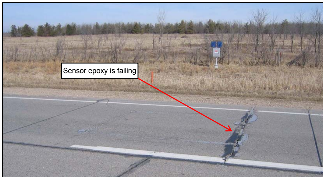
Figure 3.12: Bad Loop Sensor
