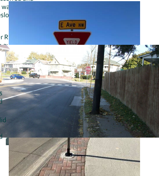
Pole not meeting offset/clear zone requirements
