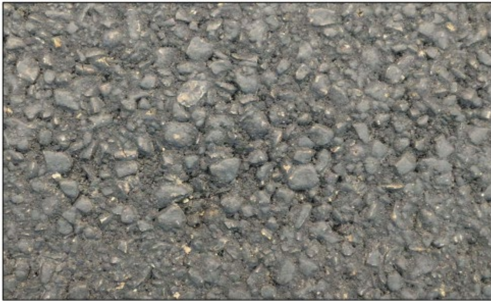
Photograph 9 - Moderate Segregation (bordering on Severe) (Close-Up)
