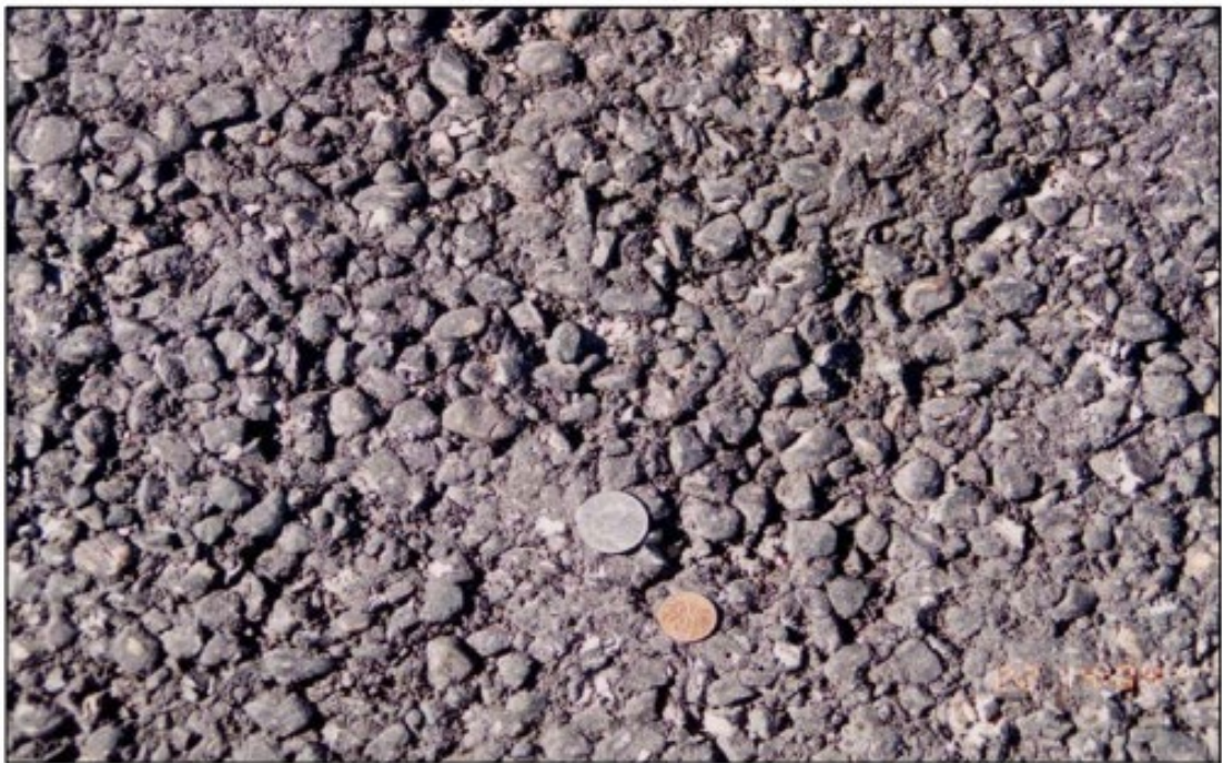
Photograph 12 - Severe Segregation (Close-Up)
