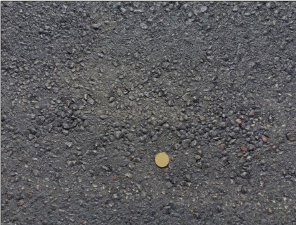
Photograph 4 - Slight Segregation (Close up)
