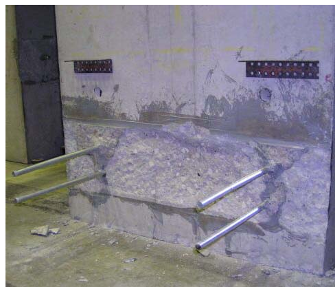
(b) Failed abutment concrete
