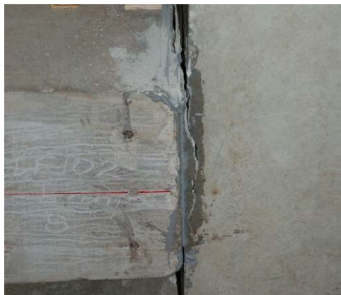
(a) Side view of the failed specimen
