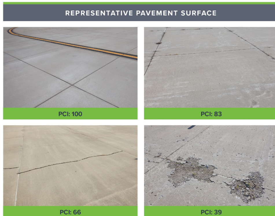
Figure 5. Visual representation of PCI scale on typical pavement surfaces.
