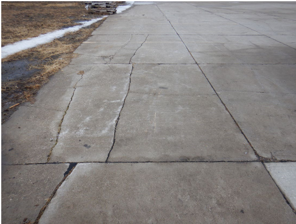
A01WC-02. Shattered Slab (Additional Sample Unit No. 17).
