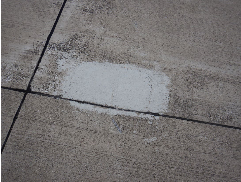
T04WC-01. Small Patching (Sample Unit No. 09).
