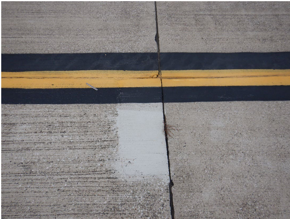
T03WC-01. Small Patching (Sample Unit No. 04).
