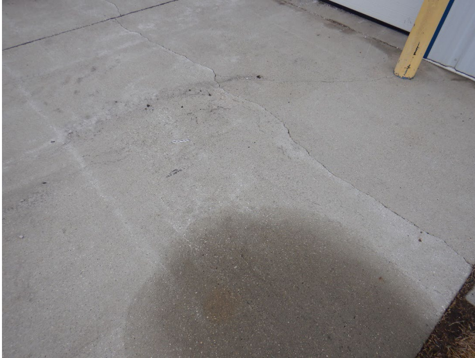
A01WC-04. LTD Cracking (Sample Unit No. 02).
