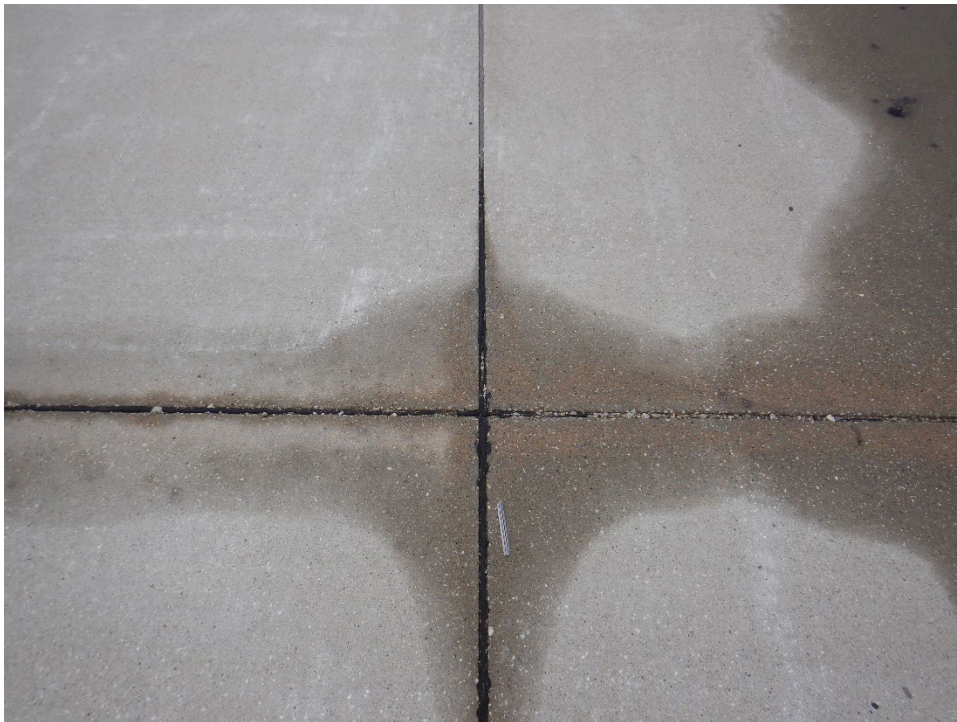
A01WC-04. Joint Seal Damage (Sample Unit No. 02).
