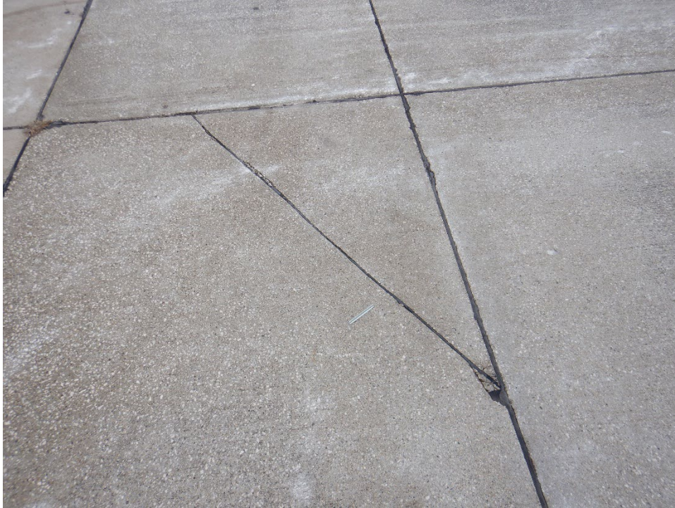
A01WC-02. LTD Cracking (Sample Unit No. 12).
