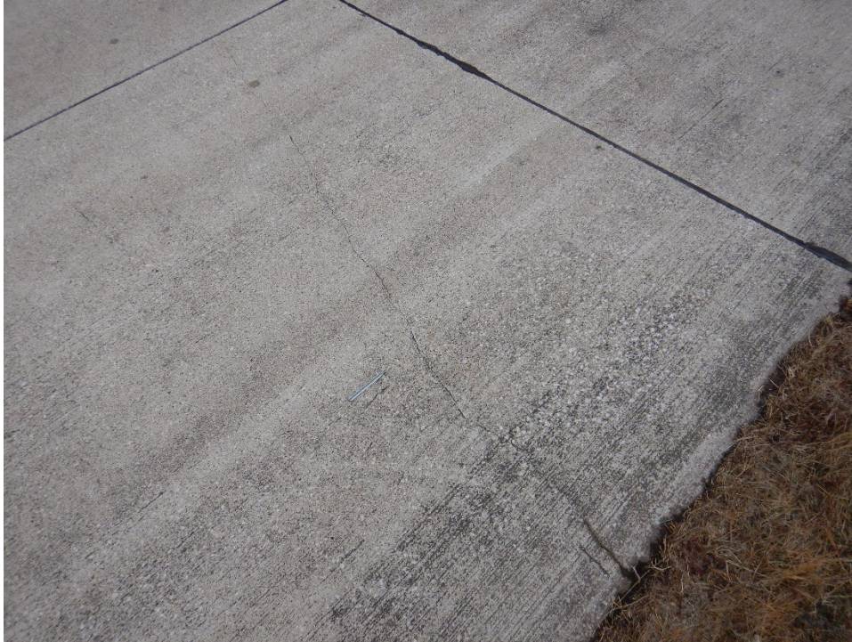
T03WC-01. LTD Cracking (Sample Unit No. 04).
