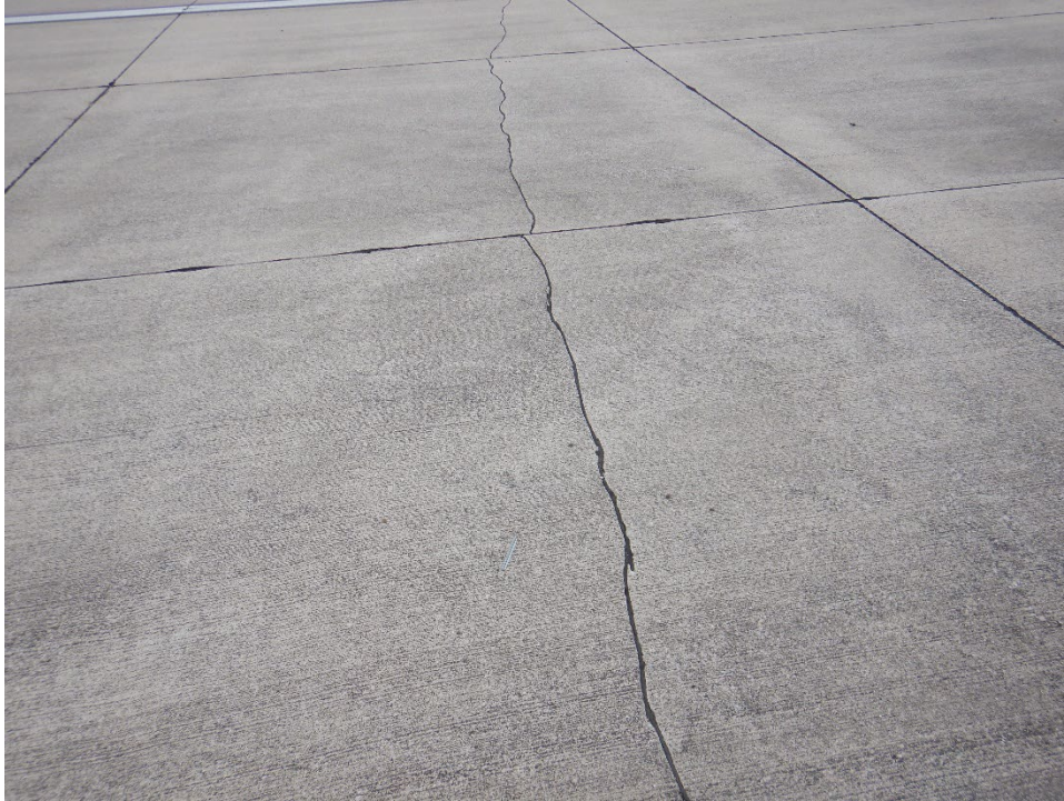
R05WC-01. LTD Cracking (Sample Unit No. 02).
