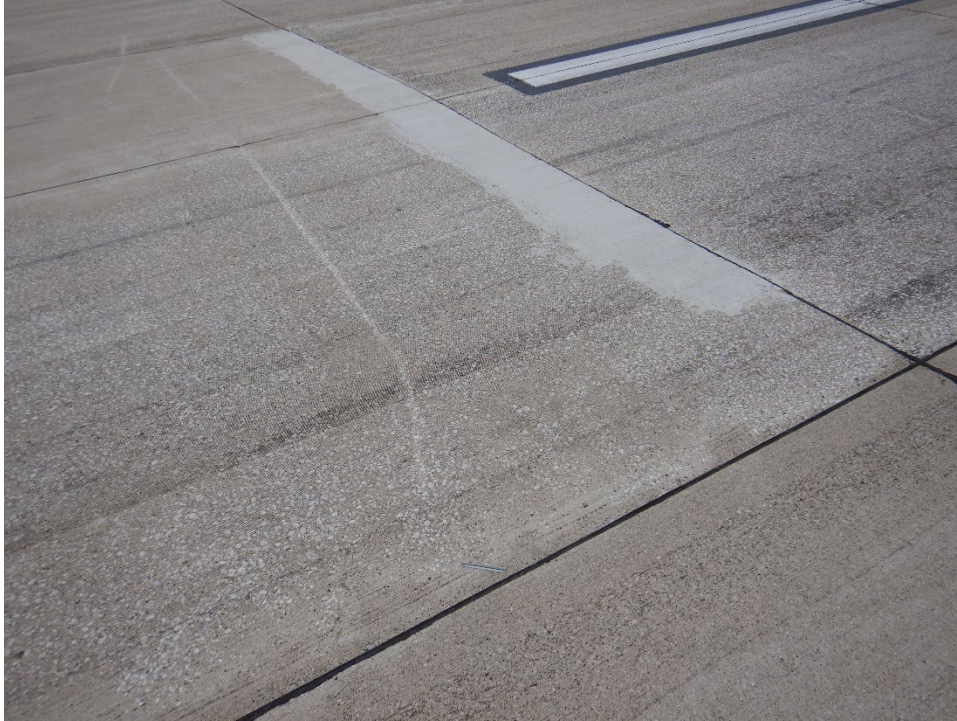
R14WC-01. Large Patching (Sample Unit No. 12).
