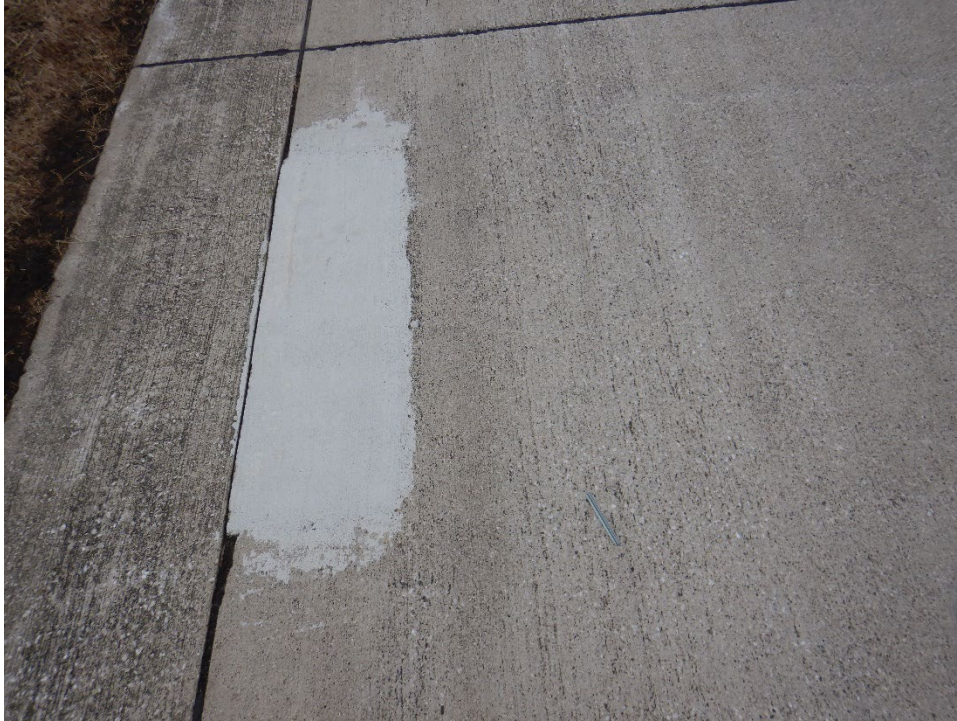
T01WC-02. Small Patching (Sample Unit No. 16).
