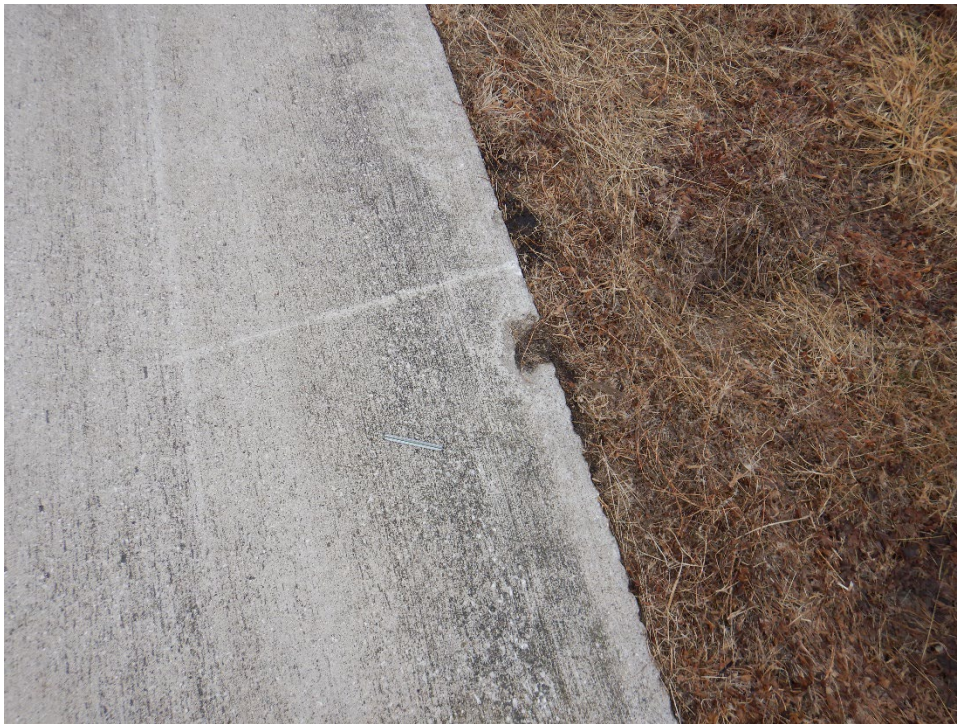
T04WC-01. Joint Spalling (Sample Unit No. 04).
