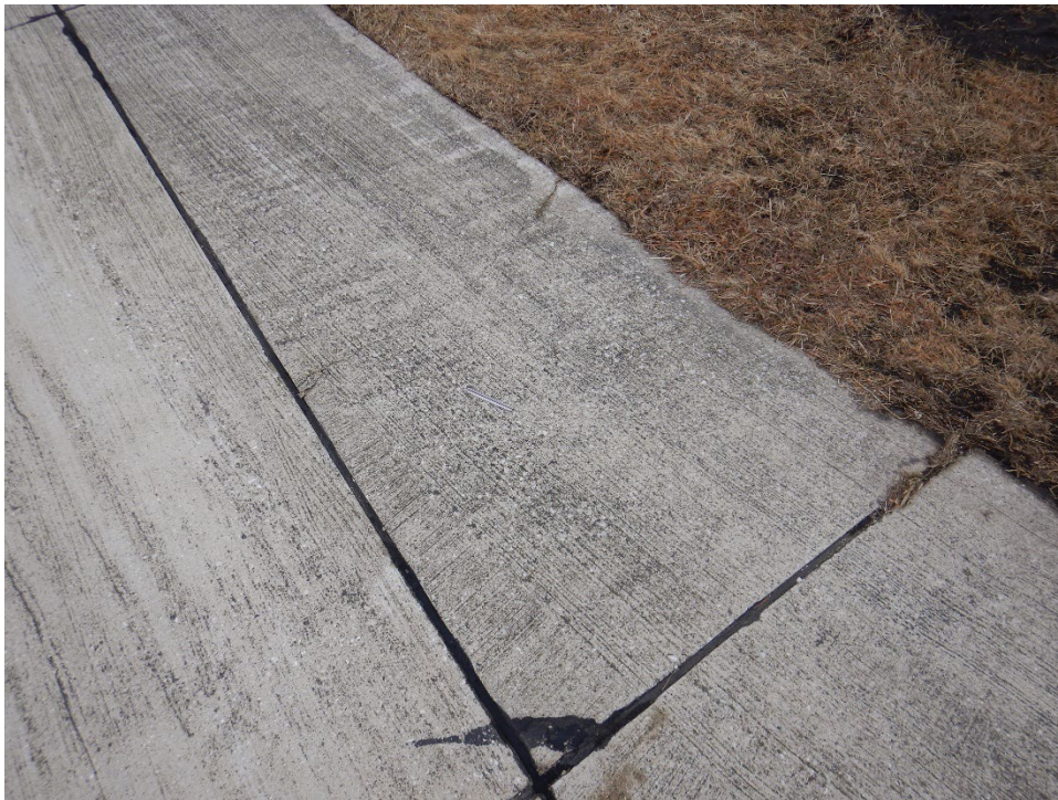
T01WC-01. LTD Cracking (Sample Unit No. 01).
