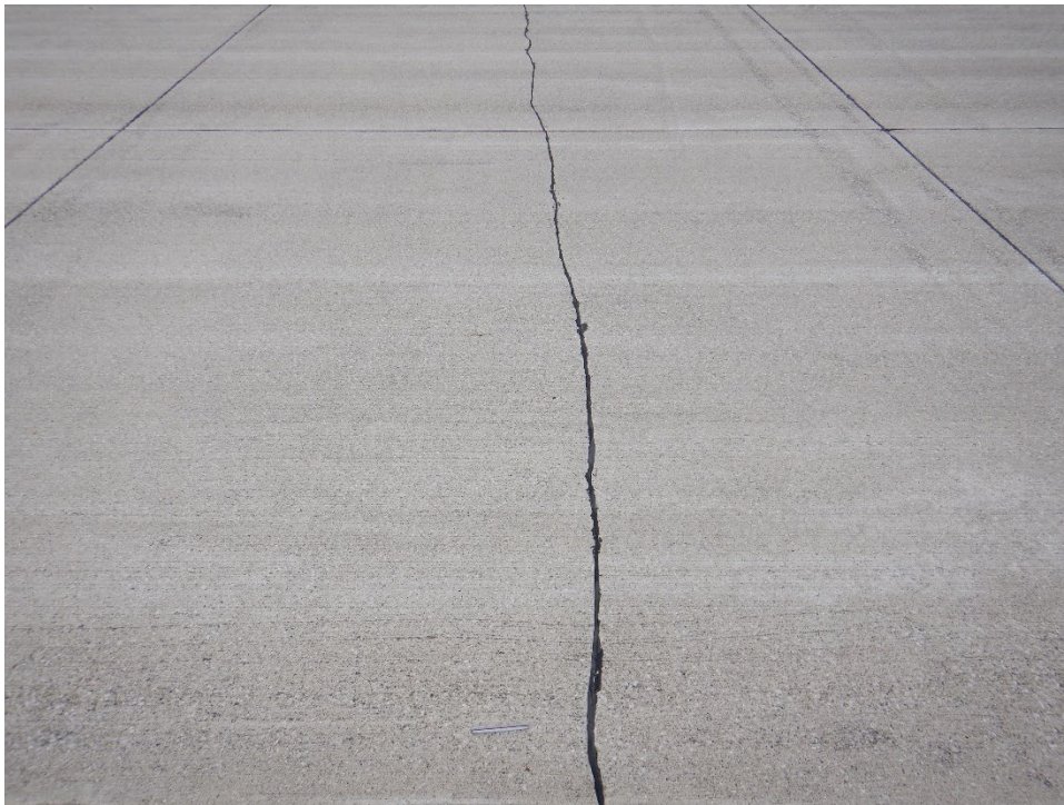
R14WC-01. LTD Cracking (Sample Unit No. 12).
