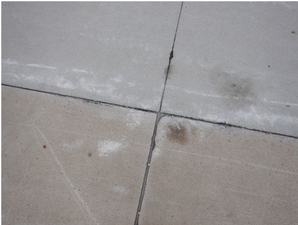
A01WC-01. Joint Seal Damage (Sample Unit No. 05).
