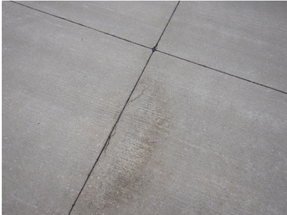
T02WC-01. Shrinkage Cracking (Sample Unit No. 11).
