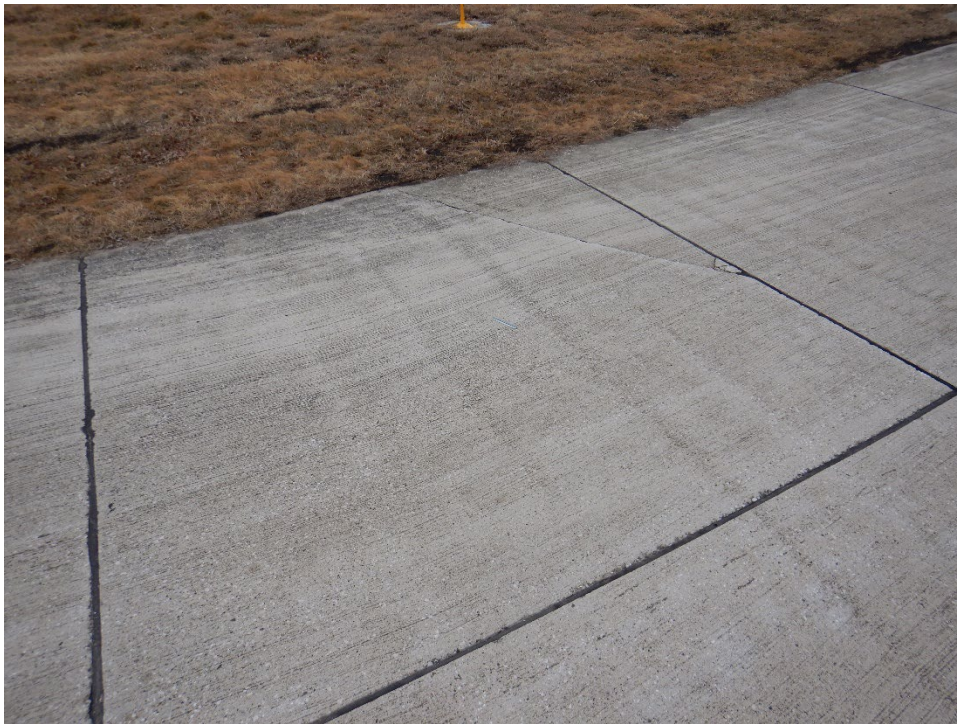
T01WC-02. LTD Cracking (Sample Unit No. 02).
