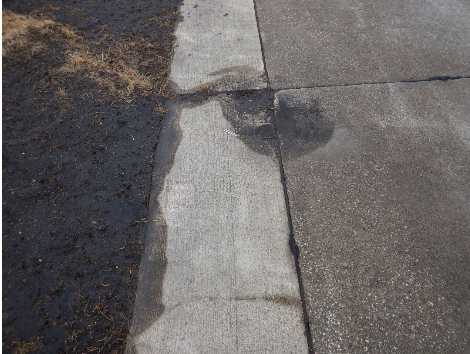
T01WC-01. Corner Break (Sample Unit No. 01).
