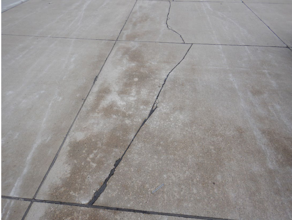
A01WC-01. LTD Cracking (Sample Unit No. 05).
