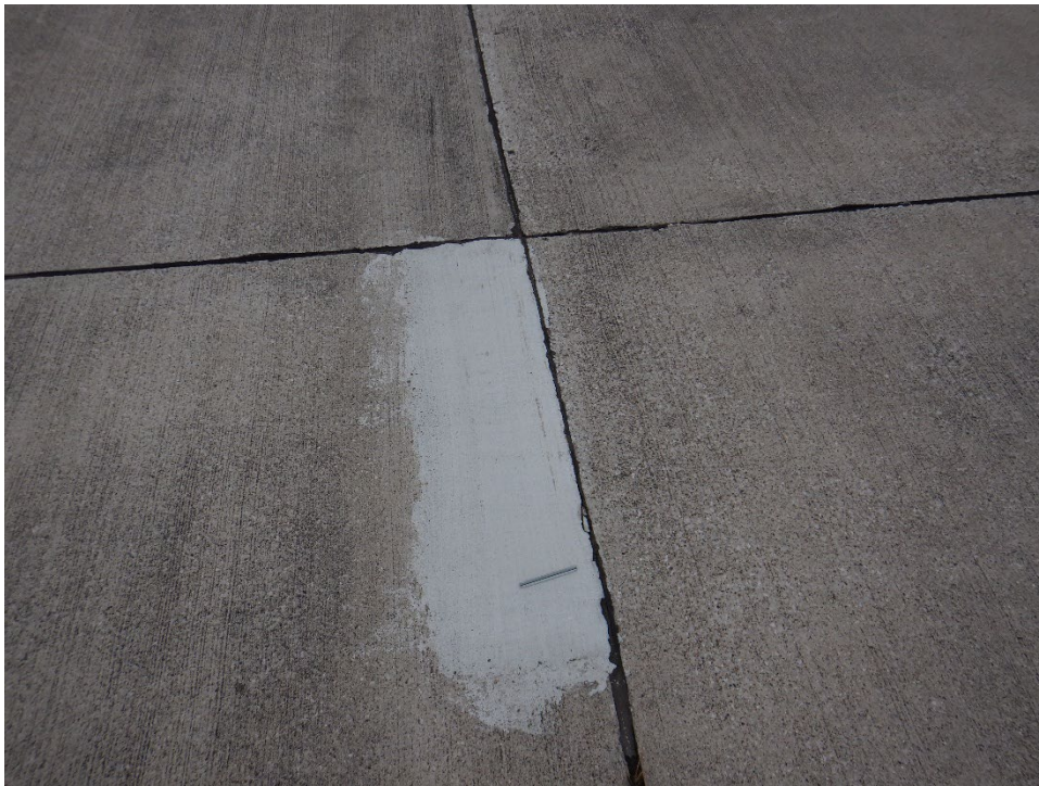
R05WC-01. Small Patching (Sample Unit No. 01).
