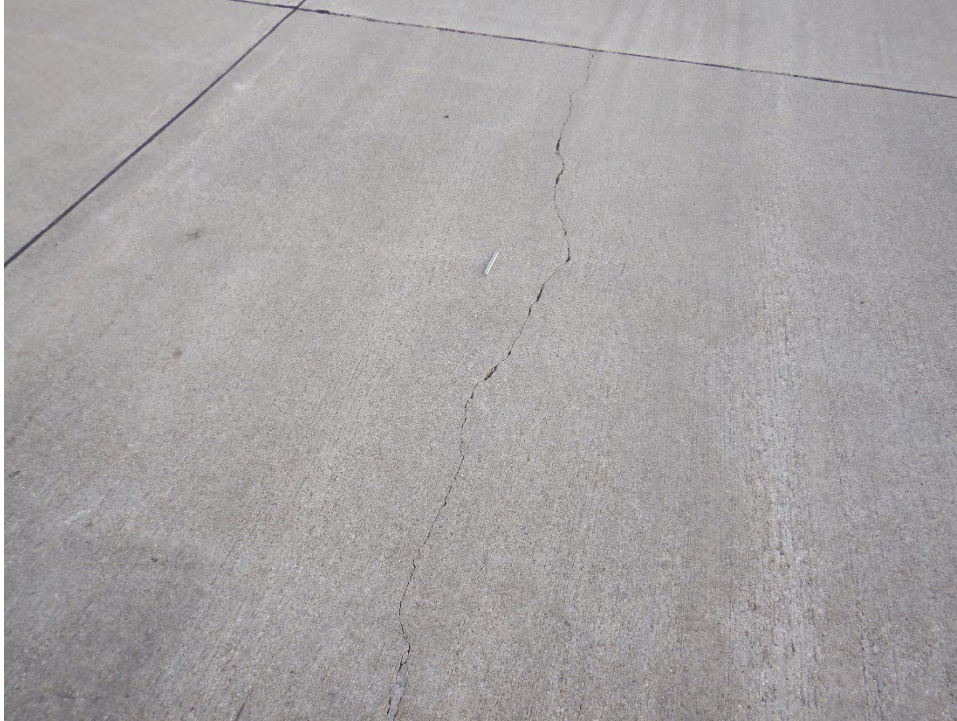
A01WV-02. LTD Cracking (Sample Unit No. 05).
