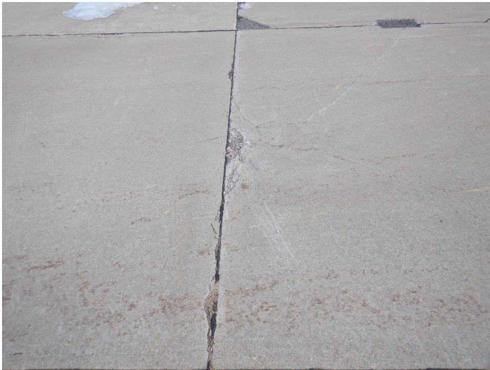
A01WV-01. Durability Cracking (Sample Unit No. 02).
