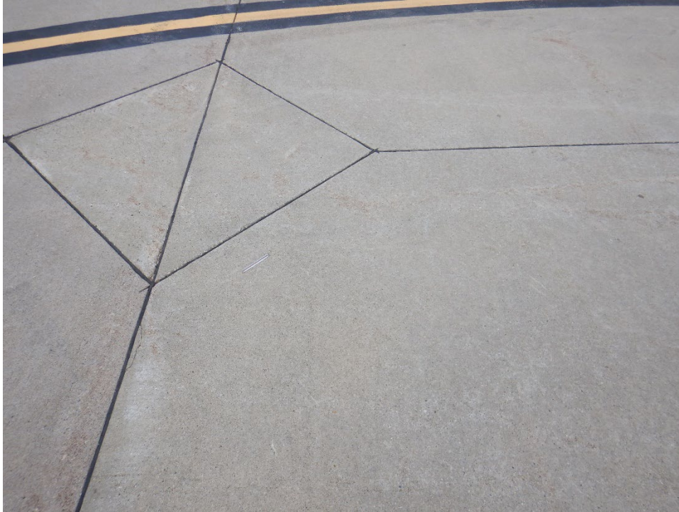
A01WV-03. Small Patching (Sample Unit No. 02).
