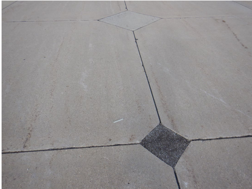
A01WV-01. Small Patching (Sample Unit No. 02).
