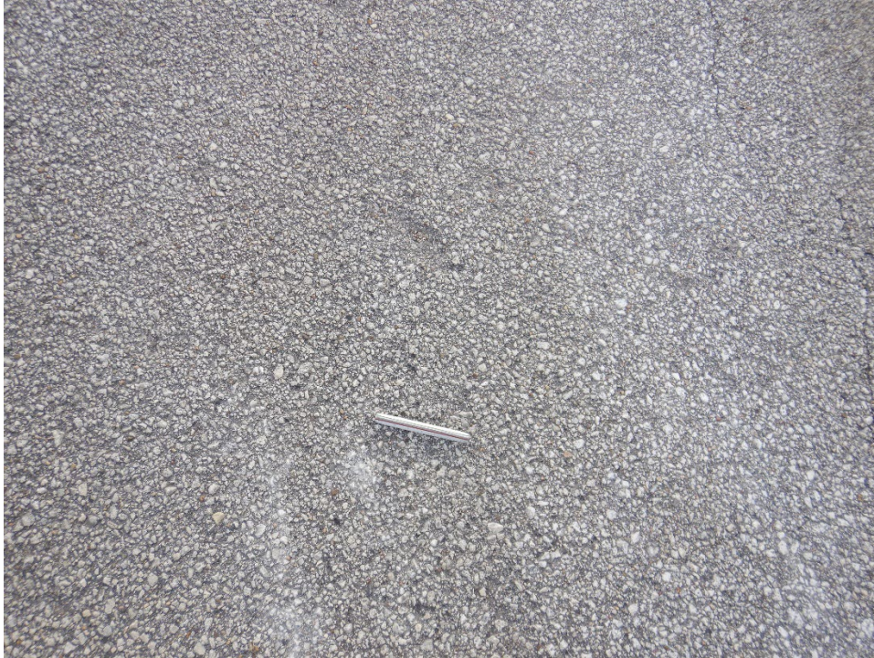
TH01WV-01. Weathering (Sample Unit No. 01).
