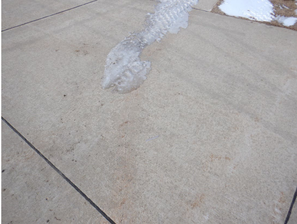
TH01WV-02. LTD Cracking (Sample Unit No. 01).
