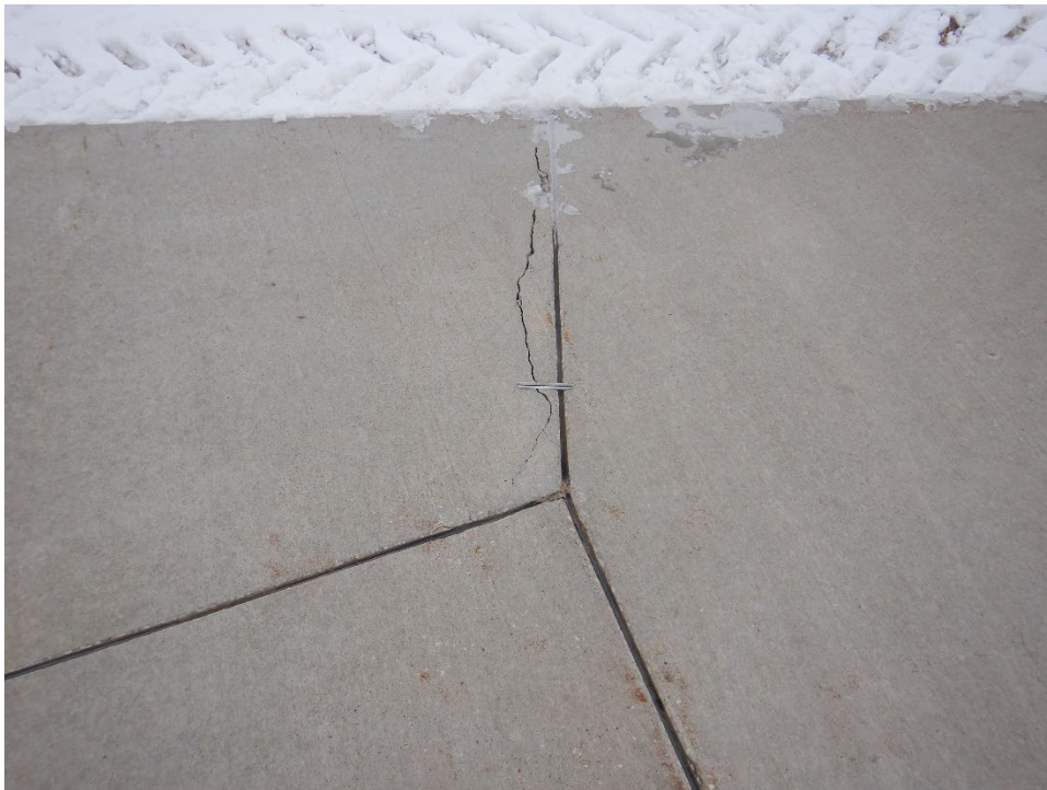
T02WV-02. Joint Spalling (Sample Unit No. 01).
