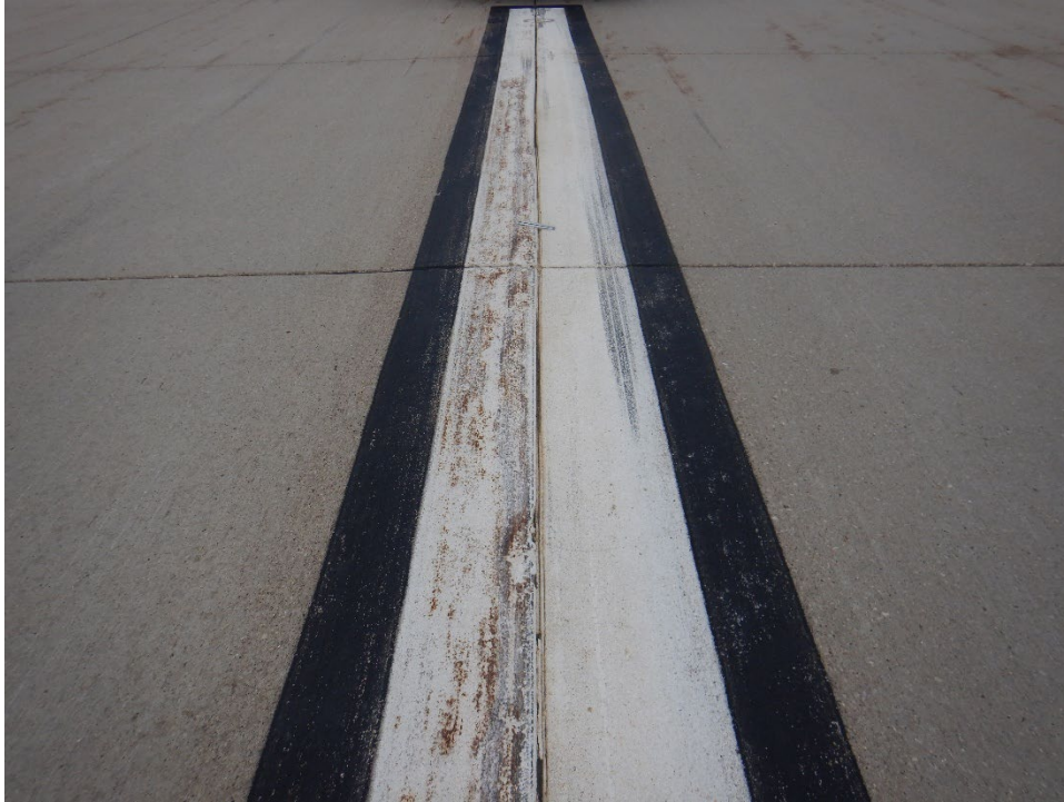
R11WV-01. Faulting (Sample Unit No. 57).
