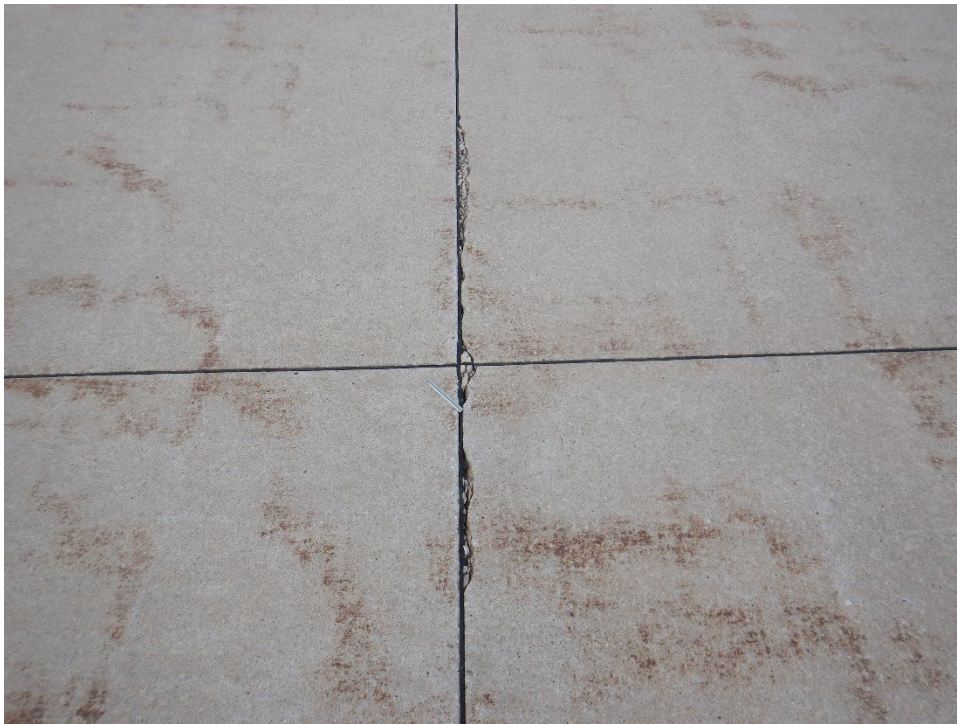
TAWV-01. Joint Seal Damage (Sample Unit No. 02).
