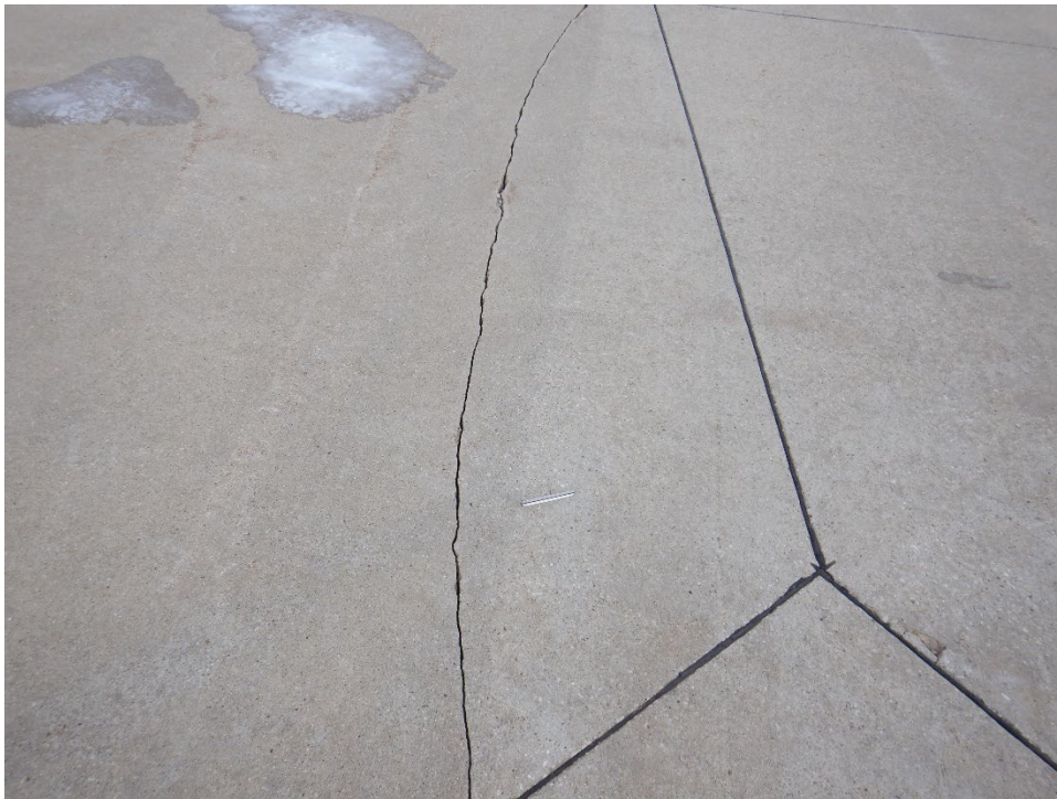
A01WV-03. LTD Cracking (Sample Unit No. 02).
