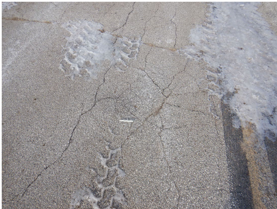
TH01WV-01. Alligator Cracking (Sample Unit No. 01).
