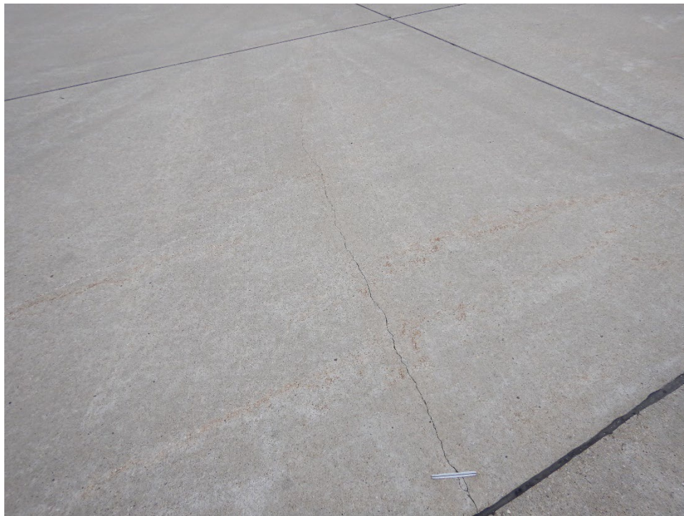
TH01WV-02. LTD Cracking (Sample Unit No. 01).
