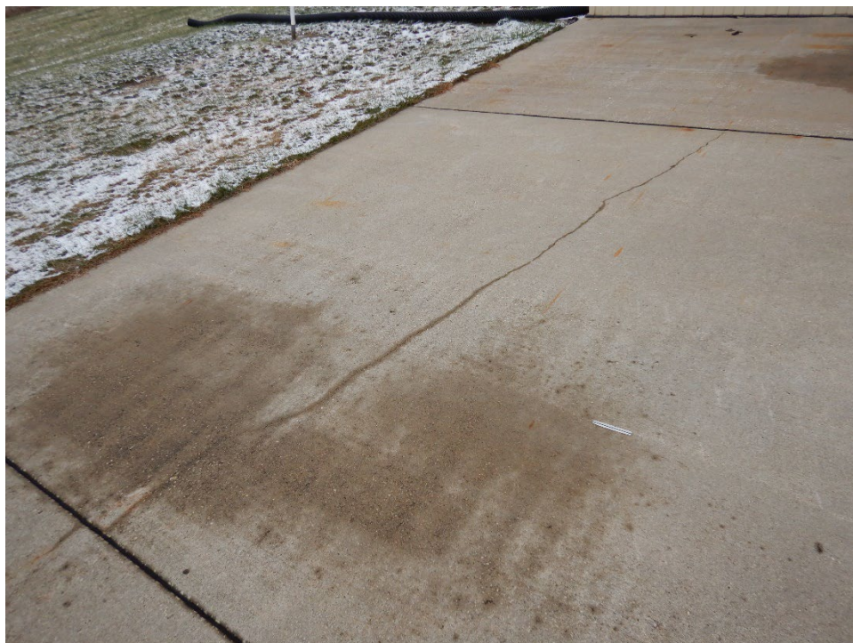
A01WV-02. LTD Cracking (Sample Unit No. 12).
