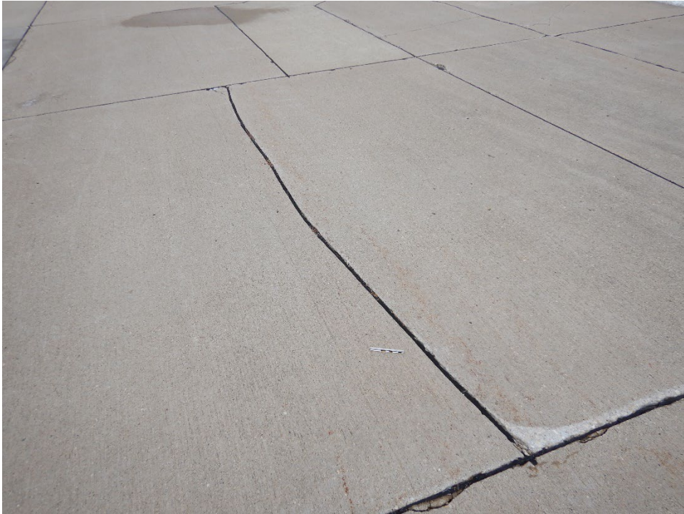
A01WV-01. LTD Cracking (Sample Unit No. 04).
