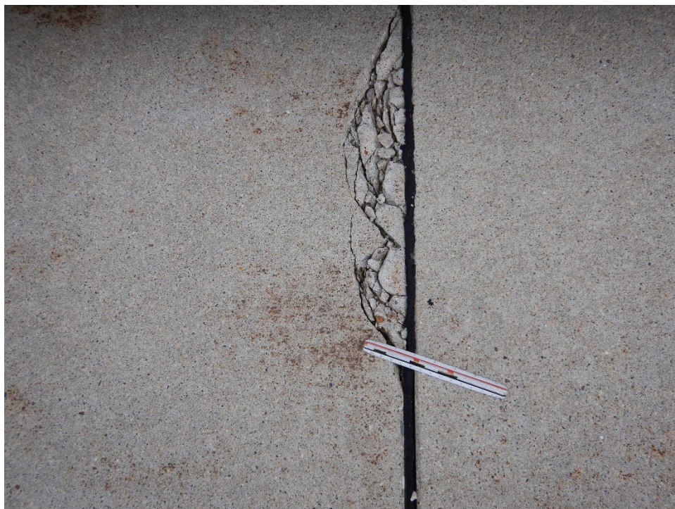
T01WV-01. Joint Spalling (Sample Unit No. 02).
