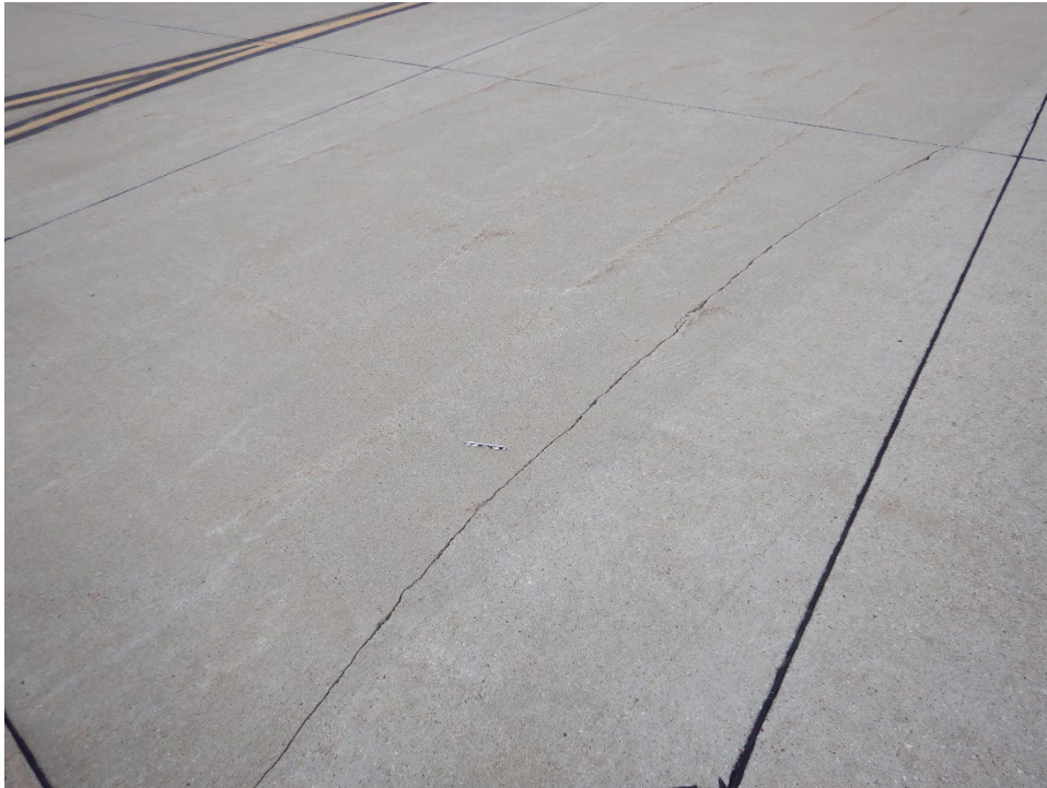
A01WV-03. LTD Cracking (Sample Unit No. 02).
