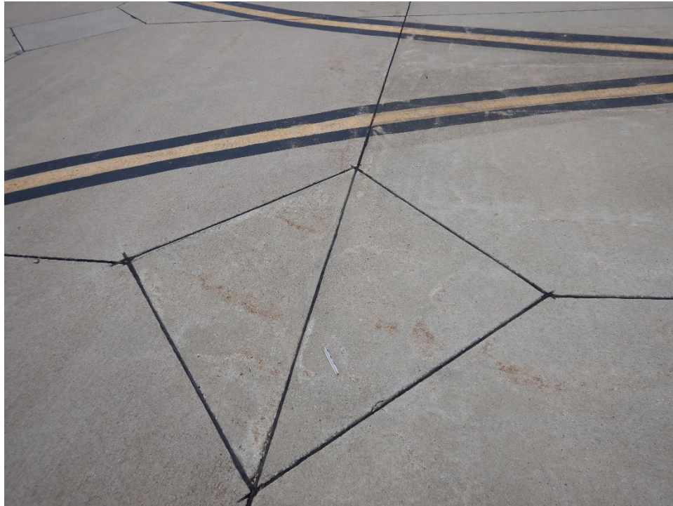
A01WV-03. Small Patching (Sample Unit No. 02).
