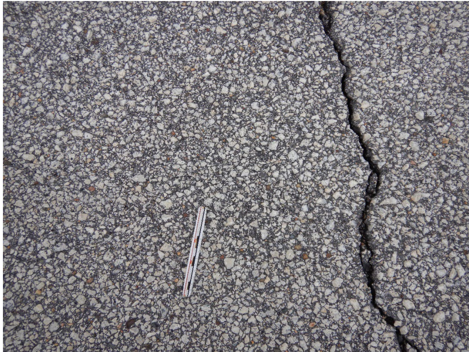
TH01WV-01. L&T Cracking (Sample Unit No. 02).
