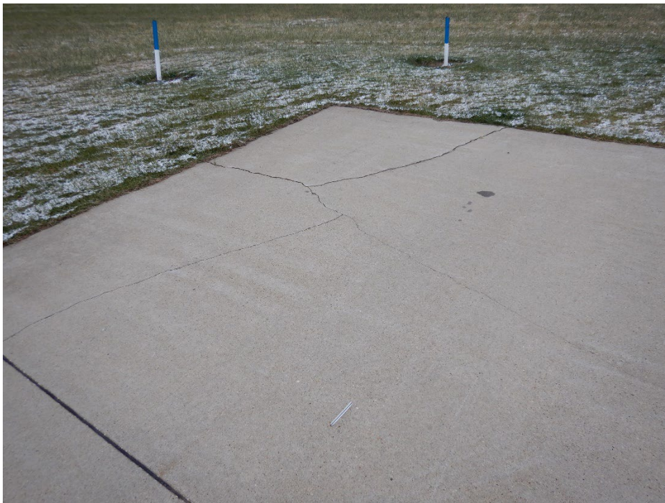
A01WV-03. Shattered Slab (Sample Unit No. 01).
