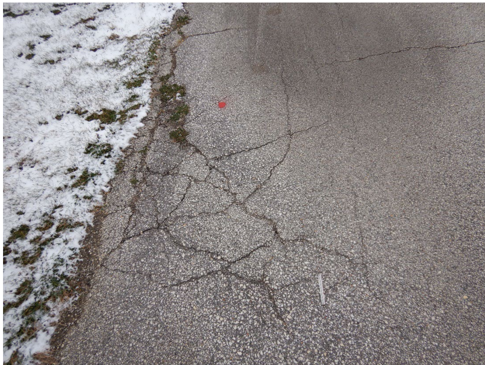
TH01WV-01. Alligator Cracking (Sample Unit No. 02).
