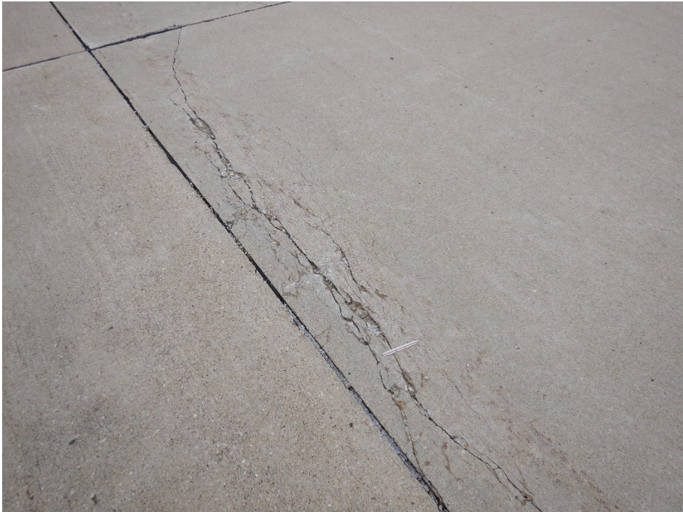
A01WV-01. Durability Cracking (Sample Unit No. 04).
