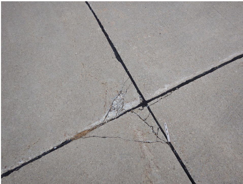
A01WV-01. Durability Cracking (Sample Unit No. 02).
