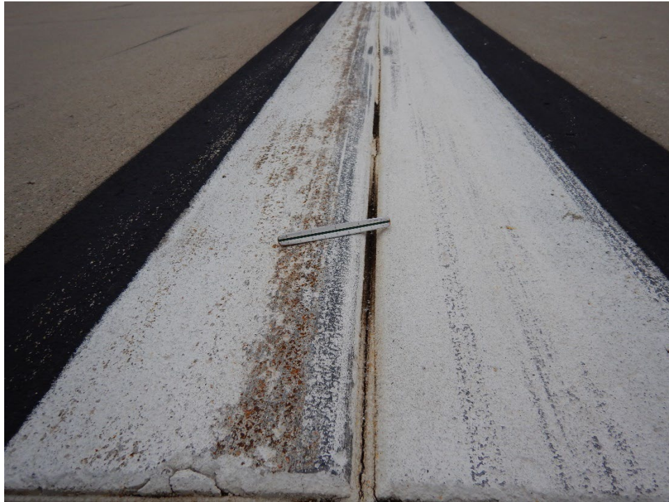
R11WV-01. Faulting (Sample Unit No. 57).
