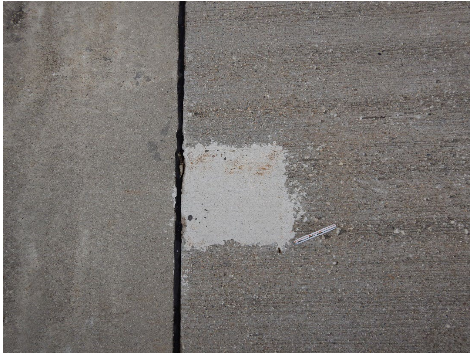
A01WV-02. Small Patching (Sample Unit No. 12).
