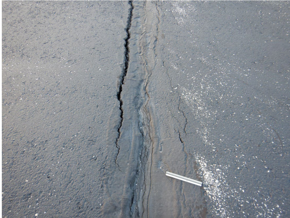
R07WK-01. L&T Cracking (Sample Unit No. 19).
