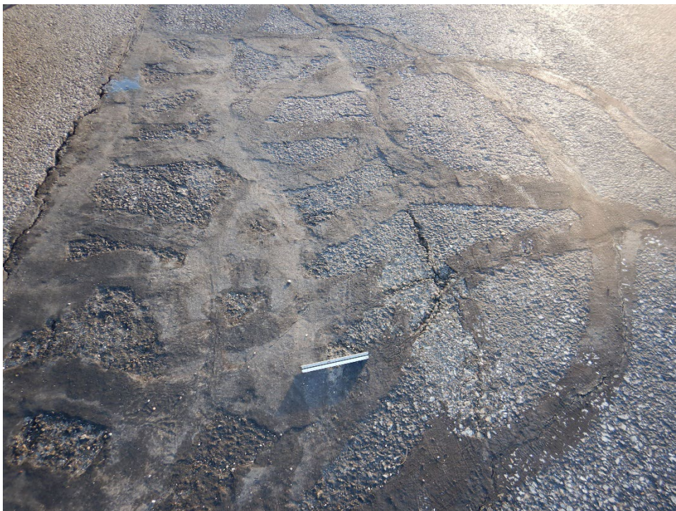
T02WK-01. Alligator Cracking (Sample Unit No. 01).
