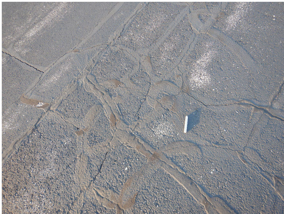
R07WK-01. Alligator Cracking (Sample Unit No. 15).
