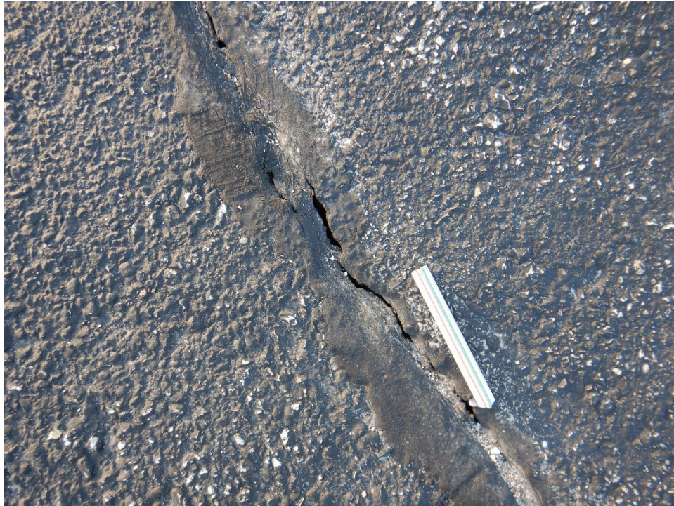
T02WK-01. L&T Cracking (Sample Unit No. 01).
