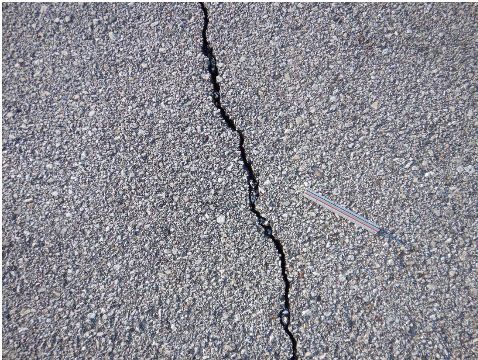
A01WK-01. L&T Cracking (Sample Unit No. 03).
