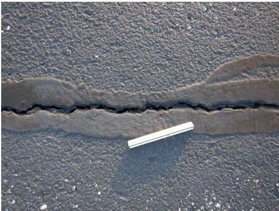
R07WK-01. L&T Cracking (Sample Unit No. 03).
