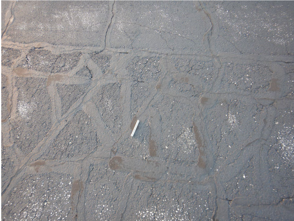
R07WK-01. Alligator Cracking (Sample Unit No. 23).
