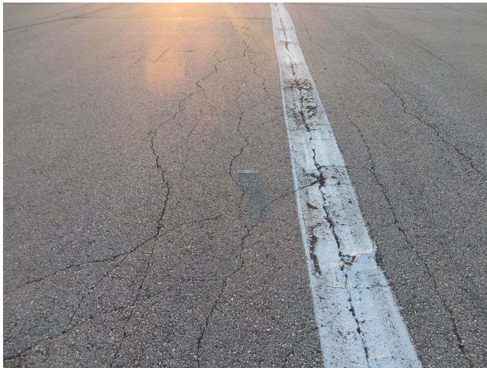
R07WK-01. Alligator Cracking (Sample Unit No. 03) (2).
