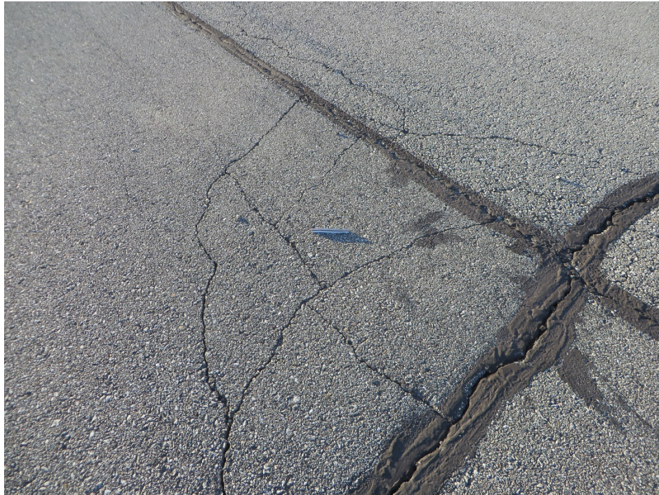
R07WK-01. Alligator Cracking (Sample Unit No. 03) (1).
