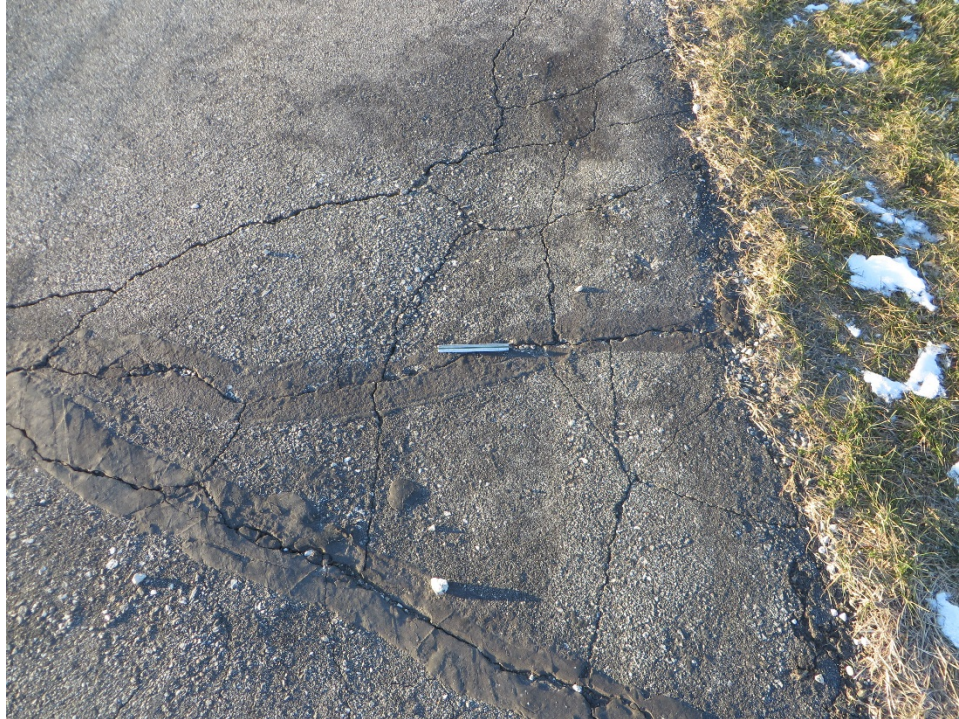
T02WK-01. Alligator Cracking (Sample Unit No. 01).
