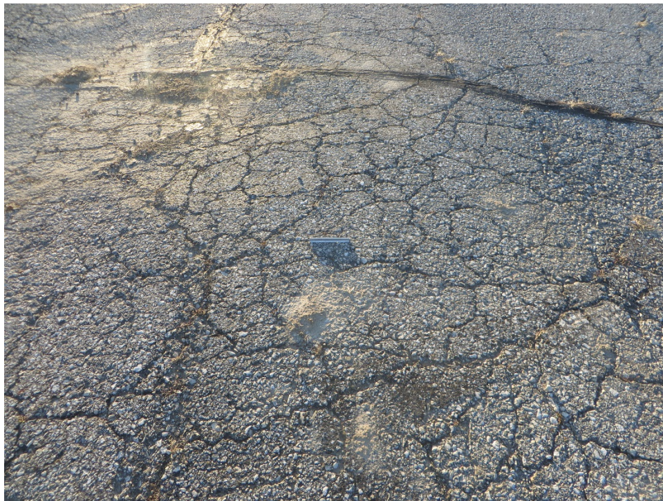
A01WK-01. Alligator Cracking (Sample Unit No. 04).
