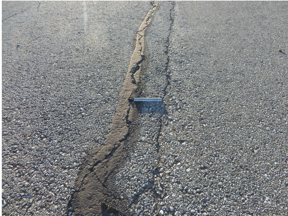
R07WK-01. L&T Cracking (Sample Unit No. 07).
