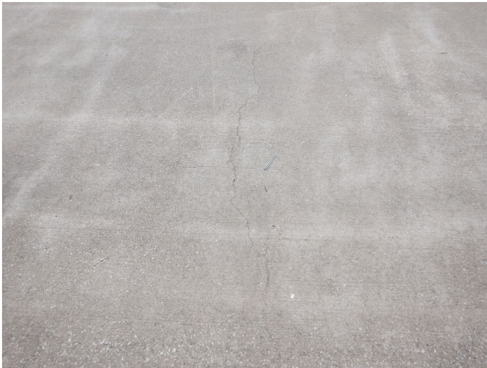
A01WA-03. LTD Cracking (Sample Unit No. 01).
