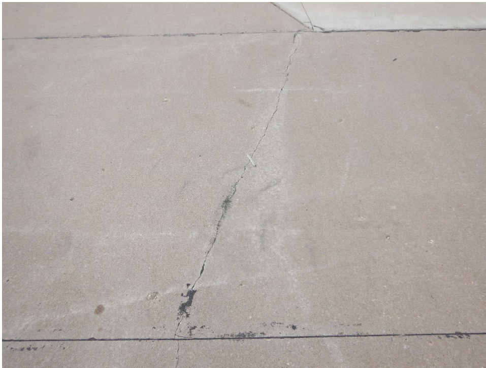
A01WA-09. LTD Cracking (Sample Unit No. 01).
