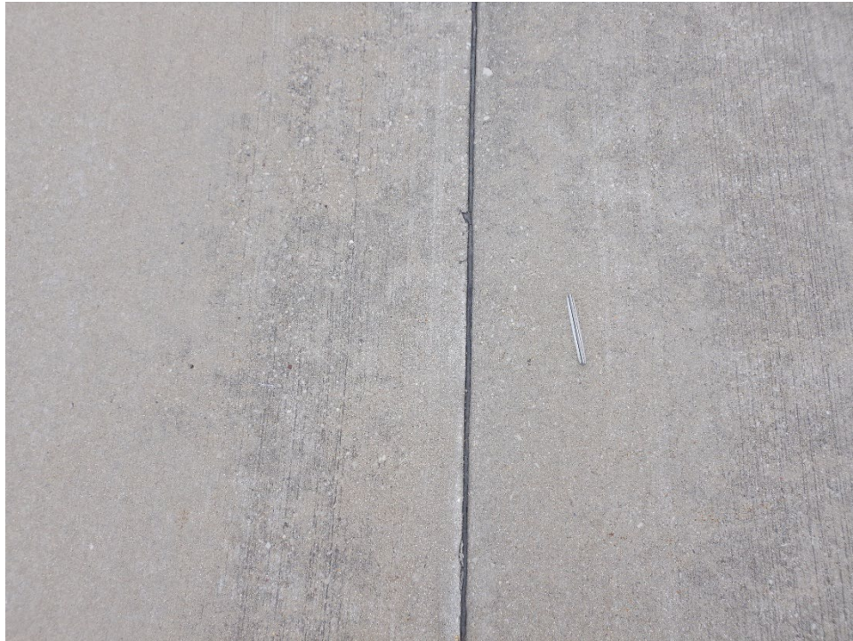
A01WA-07. Joint Seal Damage (Sample Unit No. 17).
