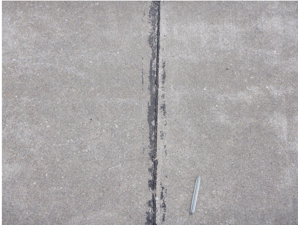
TH01WA-03. Joint Seal Damage (Sample Unit No. 01).
