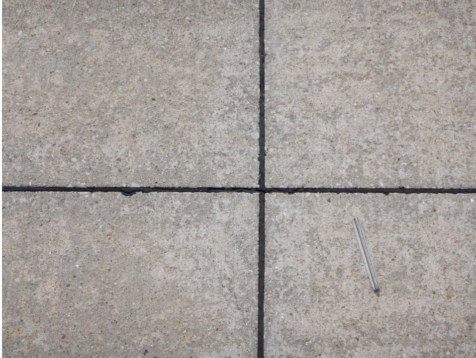
TBWA-01. Joint Seal Damage (Sample Unit No. 05).
