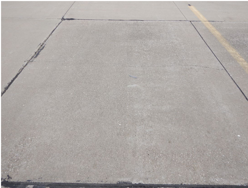
A01WA-04. LTD Cracking (Sample Unit No. 01).
