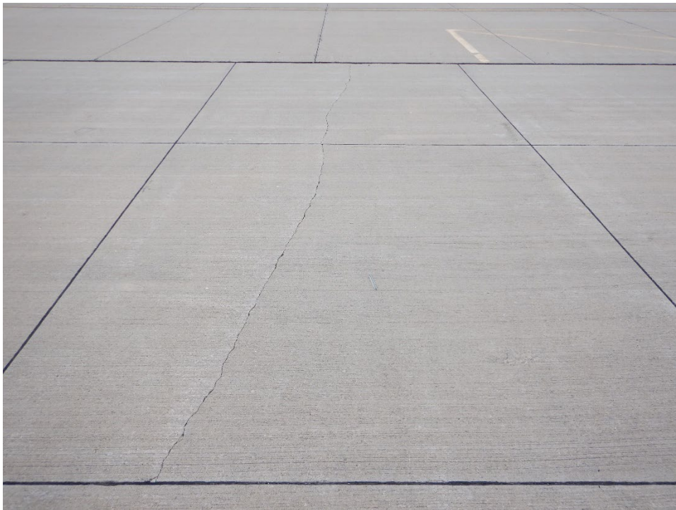
A01WA-08. LTD Cracking (Additional Sample Unit No. 03).
