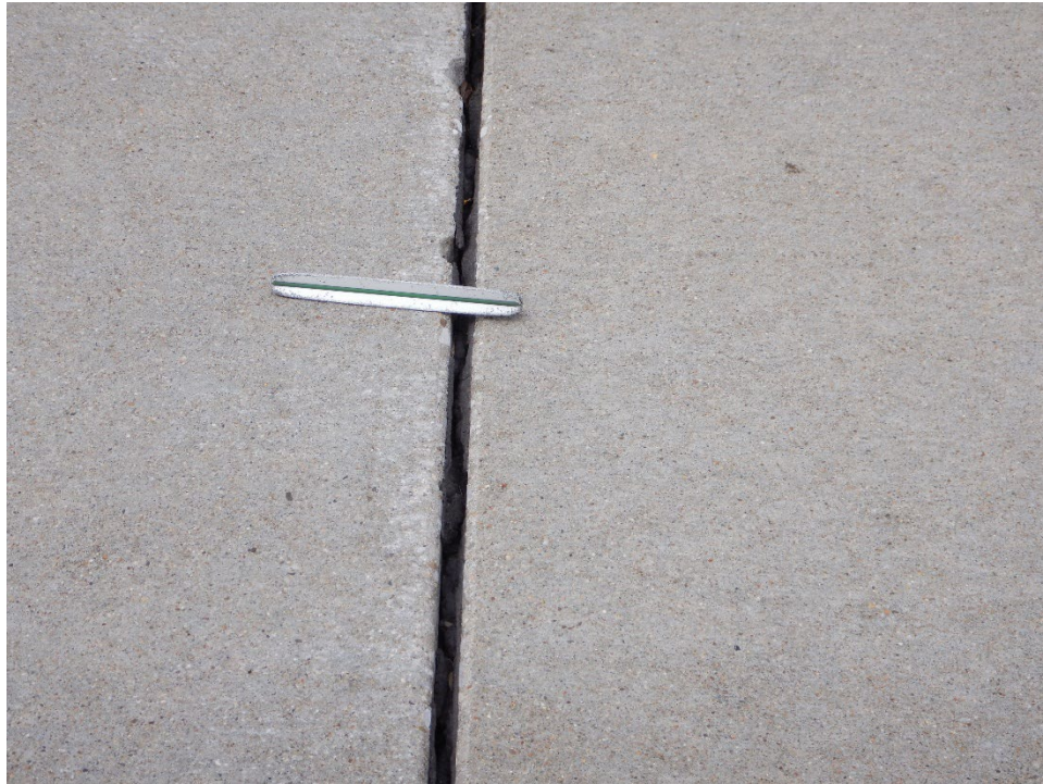
T04WA-01. Faulting (Sample Unit No. 02).
