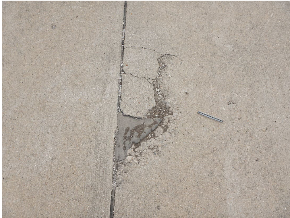
TH01WA-02. Joint Spalling (Sample Unit No. 01).
