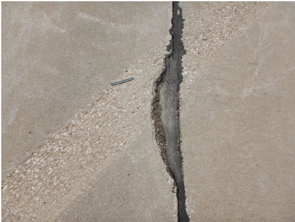
TBWA-01. Joint Spalling (Sample Unit No. 02).
