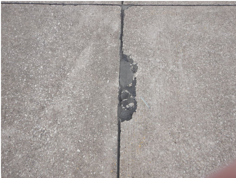
A01WA-01. Joint Spalling (Sample Unit No. 01).
