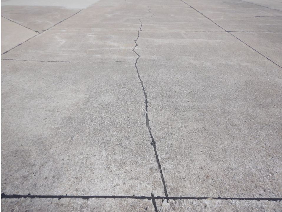
A01WA-05. LTD Cracking (Sample Unit No. 02).
