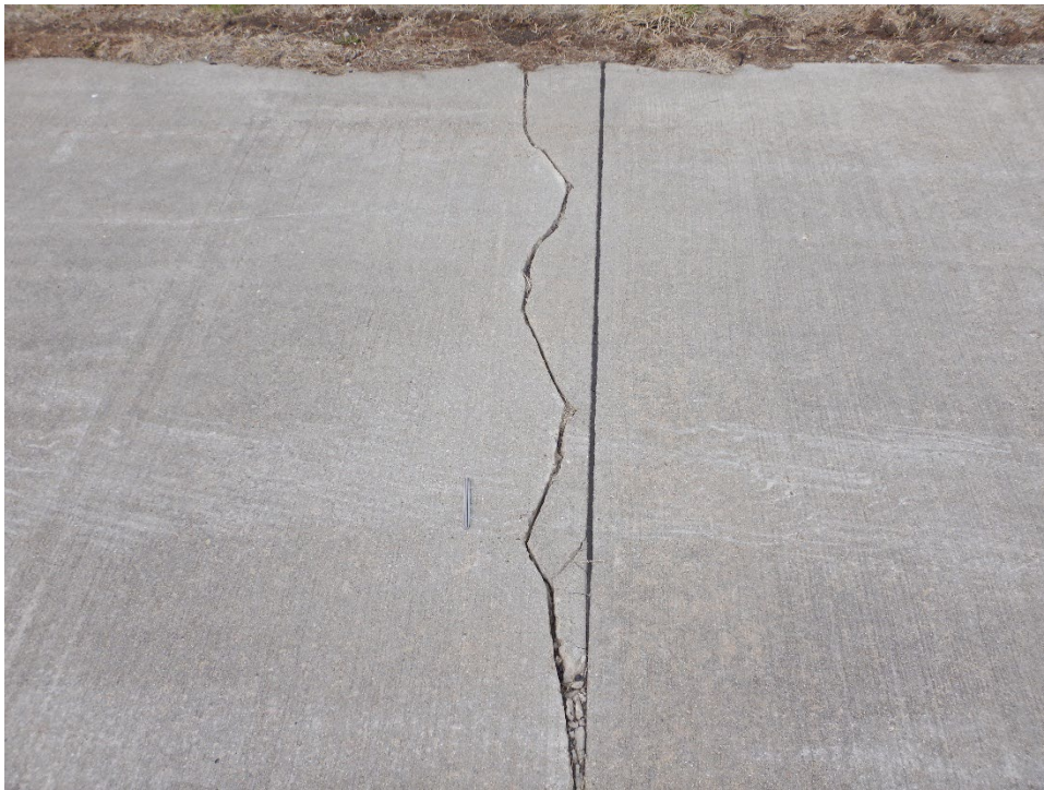
A01WA-02. Joint Spalling (Sample Unit No. 03).
