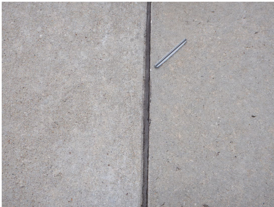
T04WA-01. Joint Seal Damage (Sample Unit No. 09).
