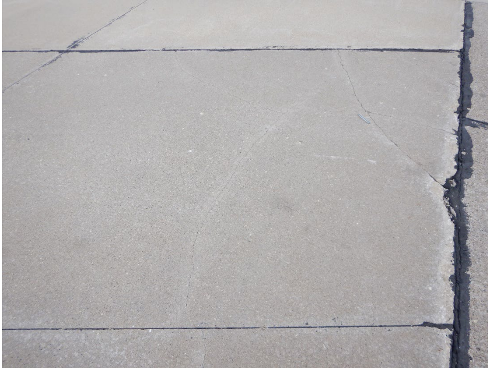
A01WA-09. Shattered Slab (Sample Unit No. 01).
