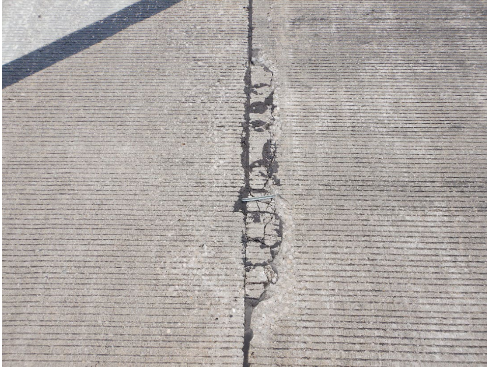
R18WA-01. Joint Spalling (Additional Sample Unit No. 08).
