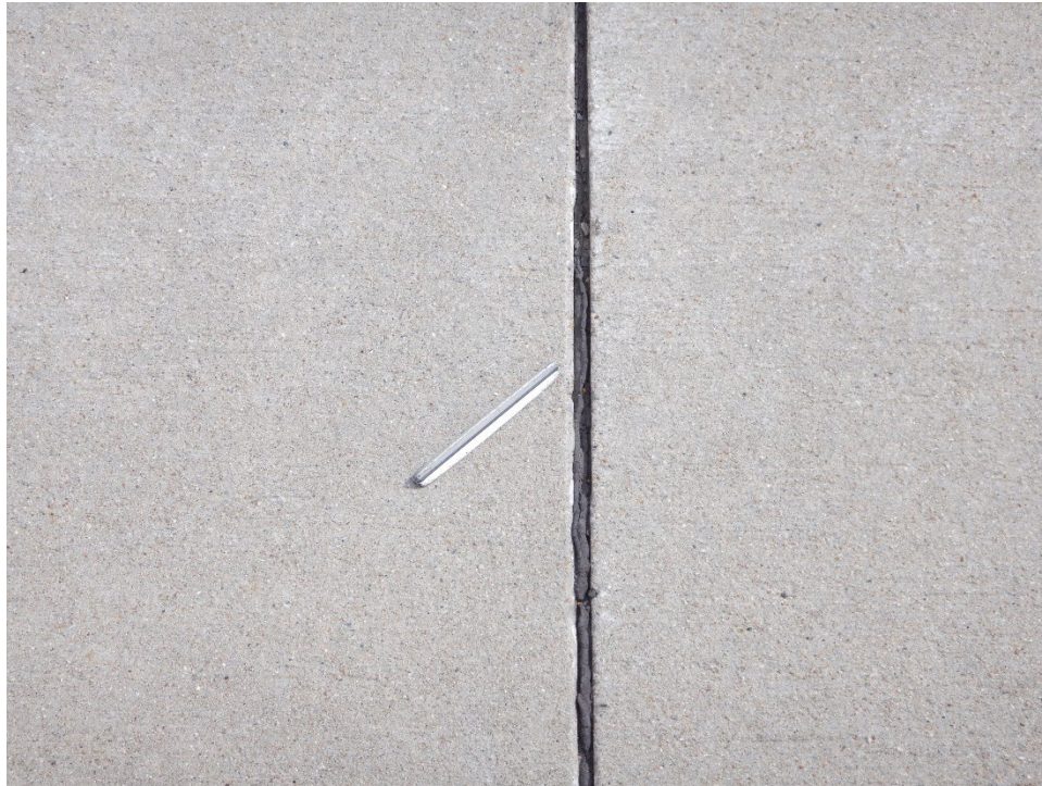
T03WA-01. Joint Seal Damage (Sample Unit No. 02).
