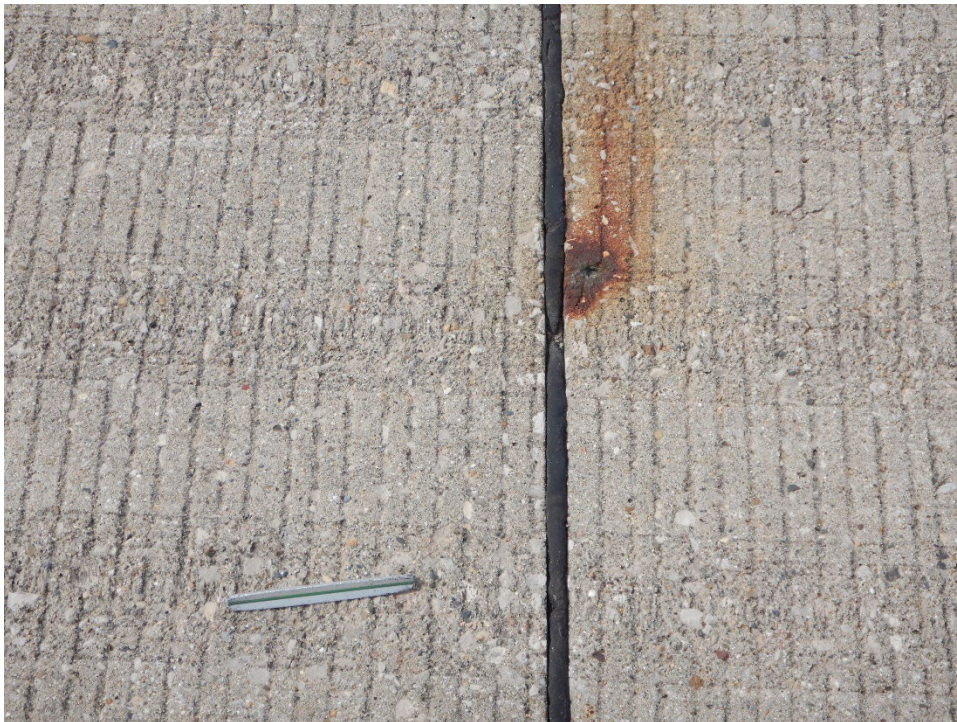
R18WA-01. Joint Seal Damage (Sample Unit No. 03).
