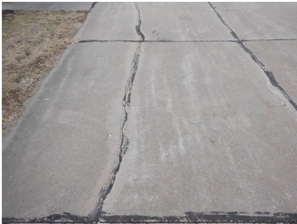
TH01WA-03. LTD Cracking (Sample Unit No. 01).
