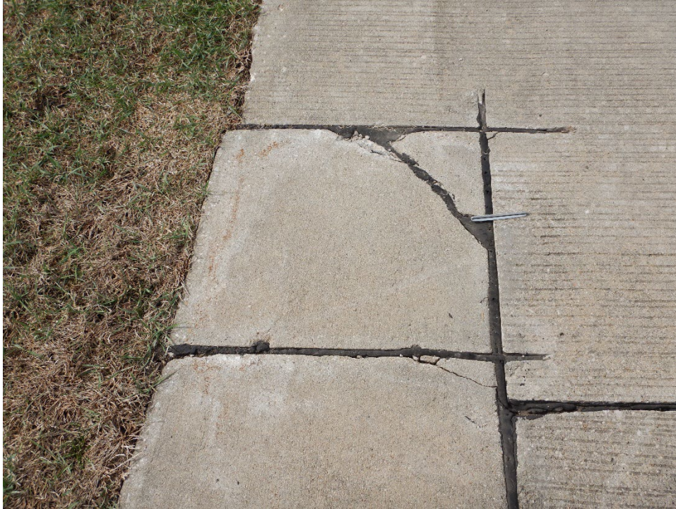
TA1WA-01. Small Patching (Sample Unit No. 02).
