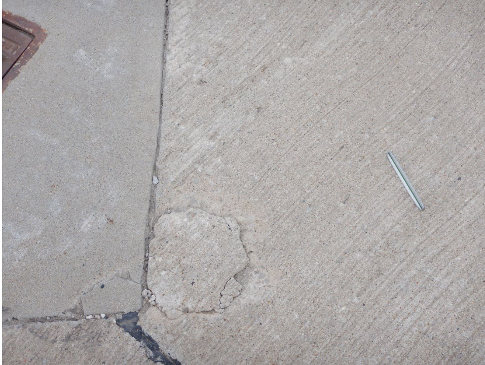
A01WA-08. Joint Spalling (Sample Unit No. 02).
