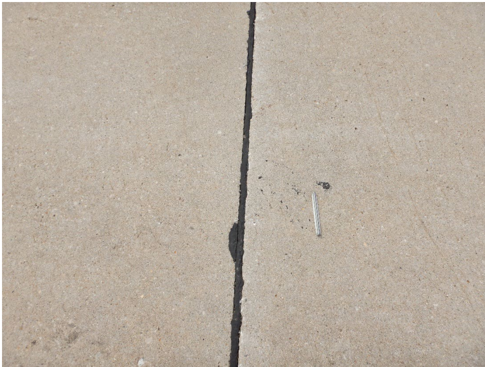
TH01WA-02. Joint Seal Damage (Sample Unit No. 02).
