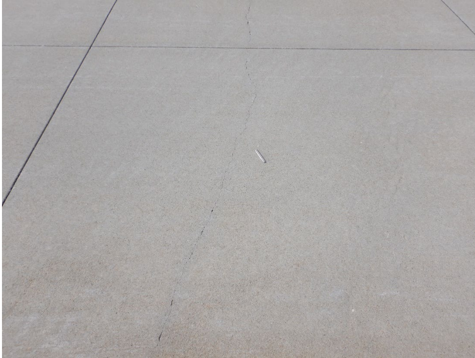
TBWA-02. LTD Cracking (Sample Unit No. 03).
