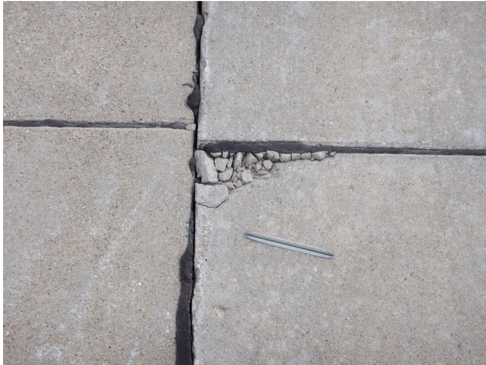
R13WA-01. Corner Spalling (Sample Unit No. 85).
