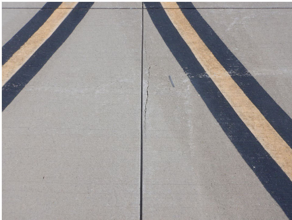
TBWA-03. Joint Spalling (Additional Sample Unit No. 12).
