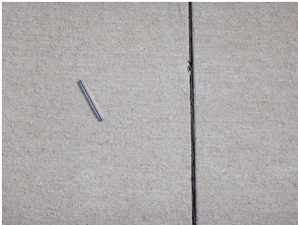
TBWA-02. Joint Seal Damage (Sample Unit No. 02).
