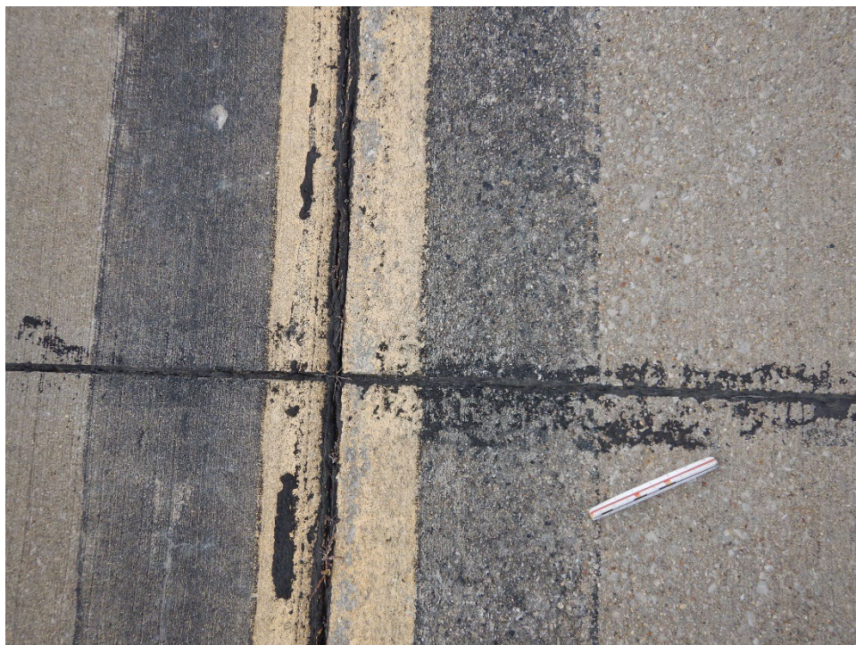
A01WA-07. Joint Seal Damage (Sample Unit No. 04).
