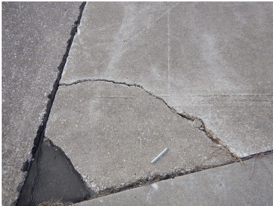
A01WA-06. Corner Break (Sample Unit No. 01).
