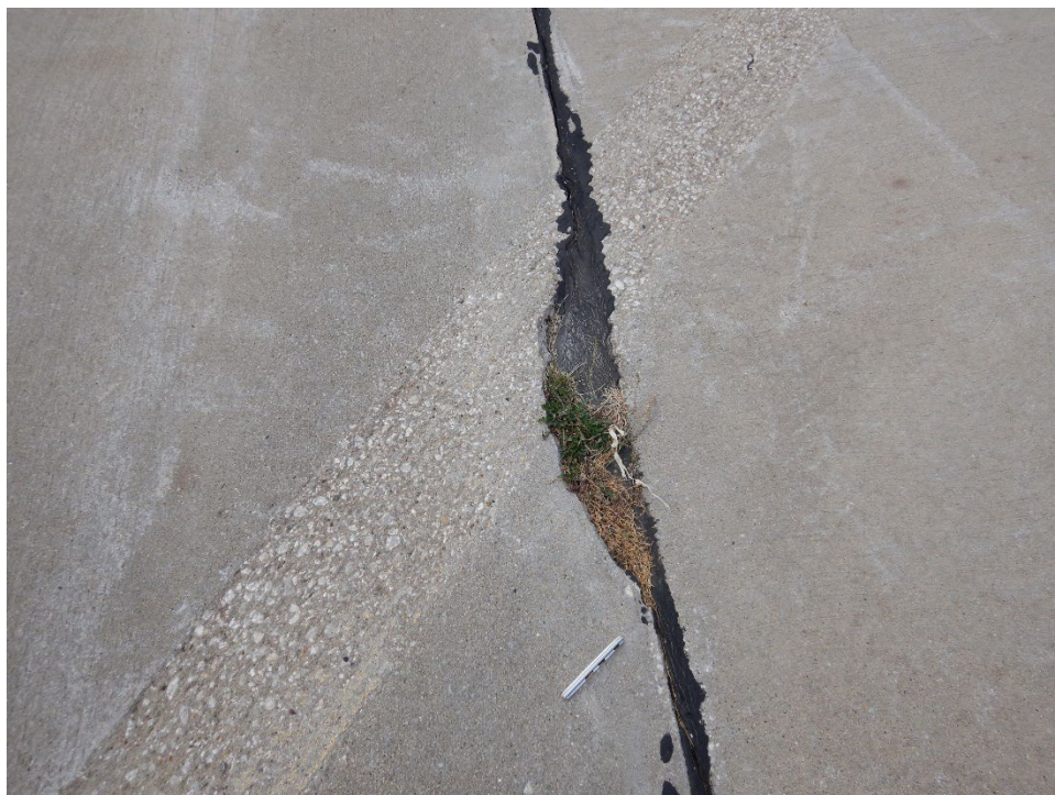
T01WA-01. Joint Spalling (Sample Unit No. 02).
