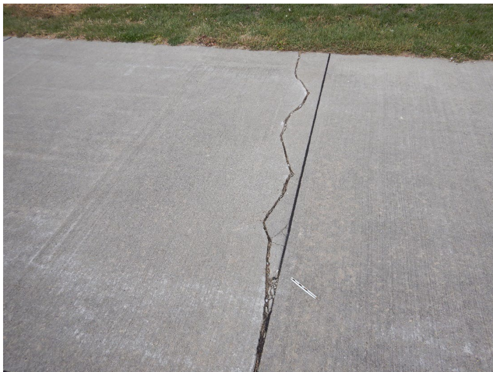
A01WA-02. Joint Spalling (Sample Unit No. 03).
