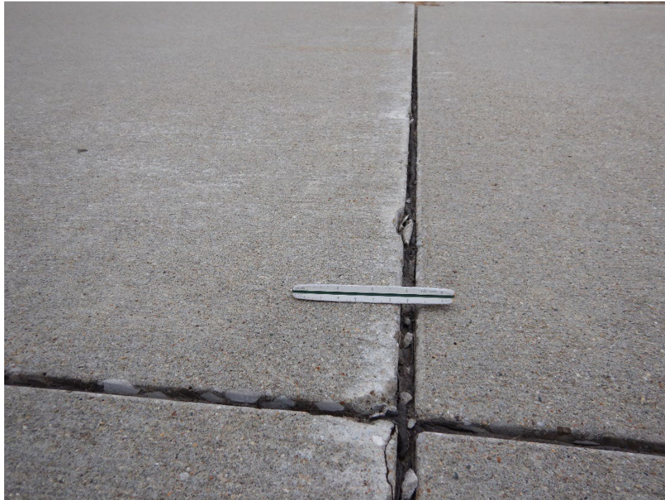
T04WA-01. Faulting (Sample Unit No. 02).
