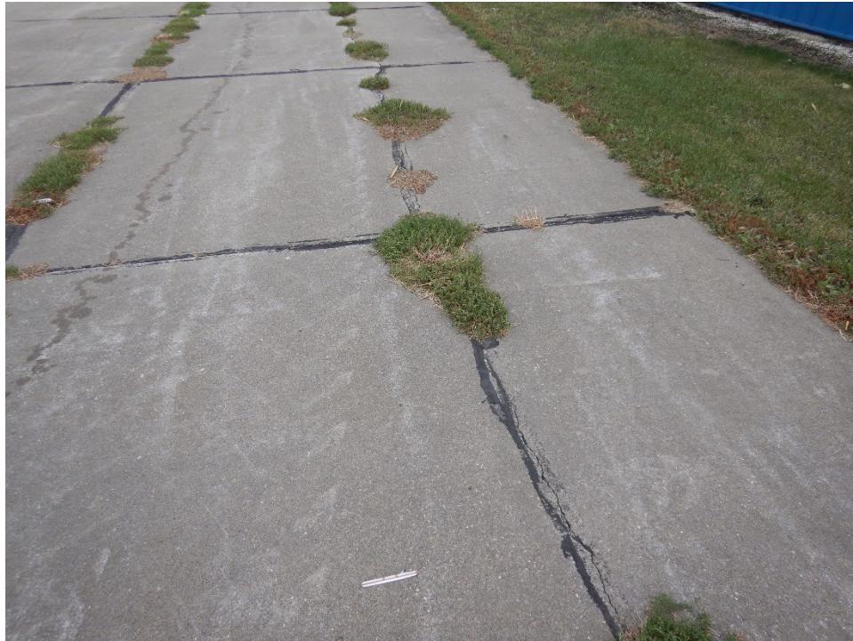
TH01WA-03. LTD Cracking (Sample Unit No. 01).
