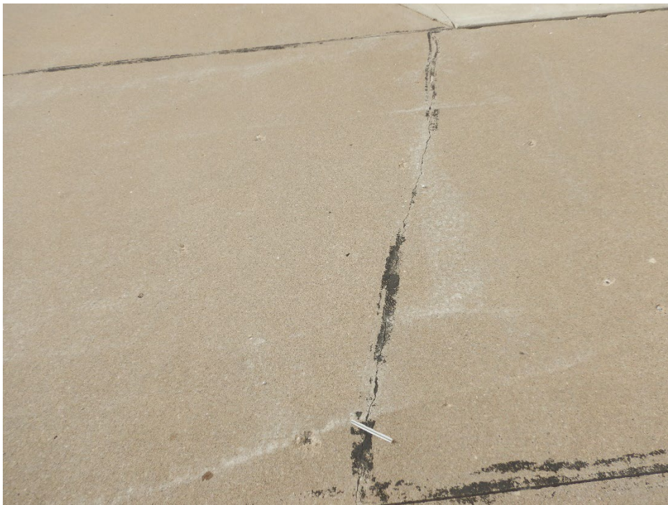
A01WA-09. LTD Cracking (Sample Unit No. 01).
