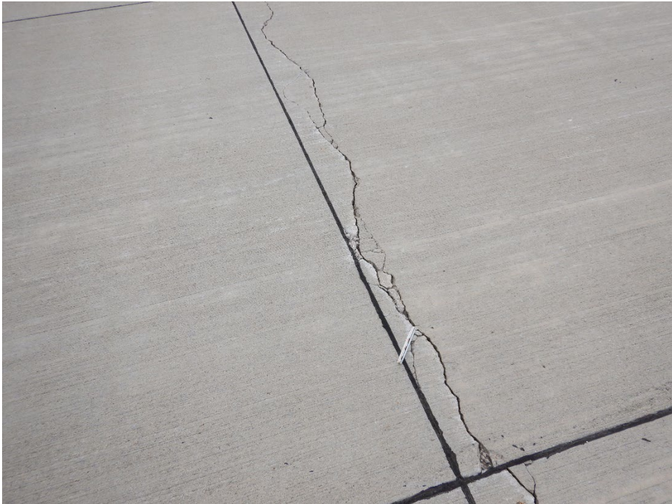
A01WA-08. Joint Spalling (Sample Unit No. 05).
