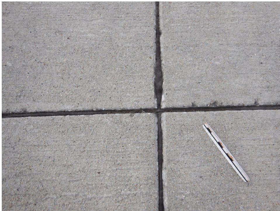
R13WA-01. Joint Seal Damage (Sample Unit No. 15).
