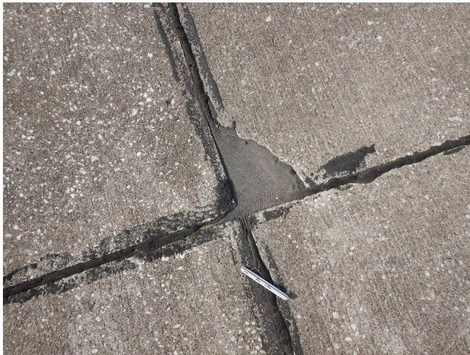
A01WA-01. Corner Spalling (Sample Unit No. 02).
