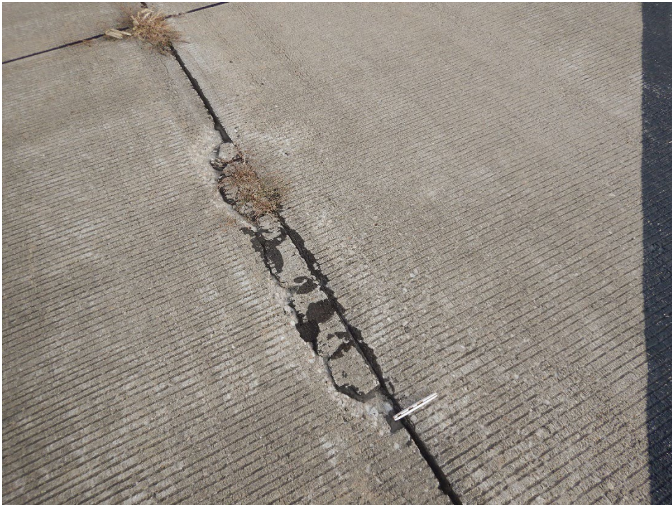
R18WA-01. Joint Spalling (Additional Sample Unit No. 08).
