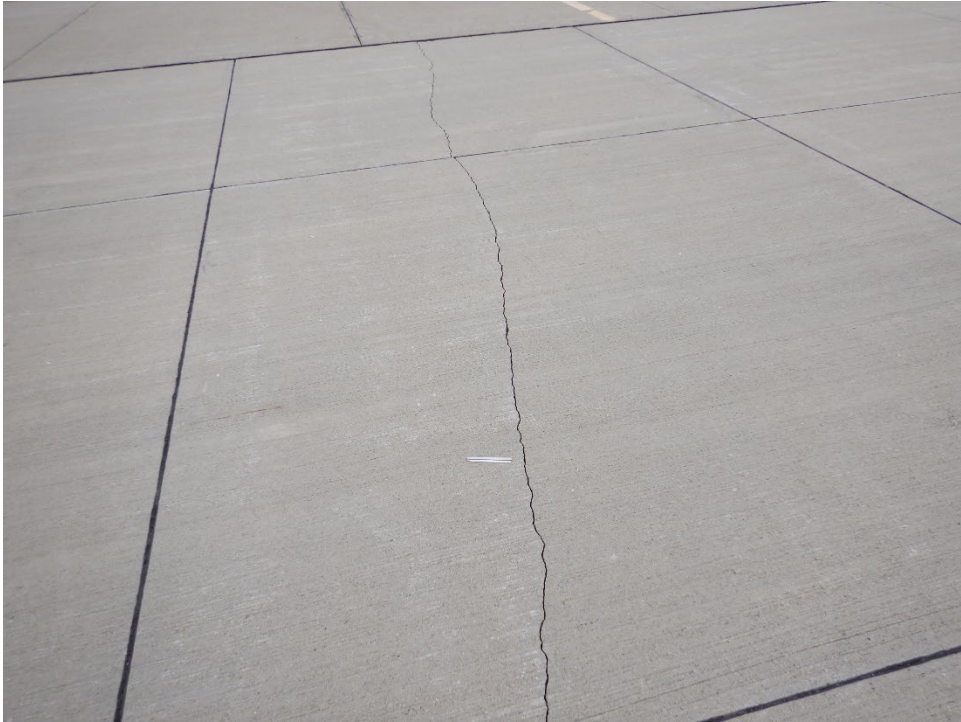
A01WA-08. LTD Cracking (Additional Sample Unit No. 03).
