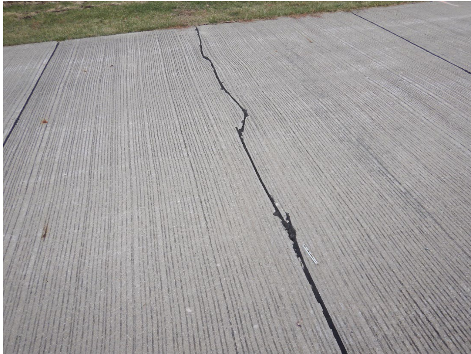
T02WA-01. LTD Cracking (Sample Unit No. 06).
