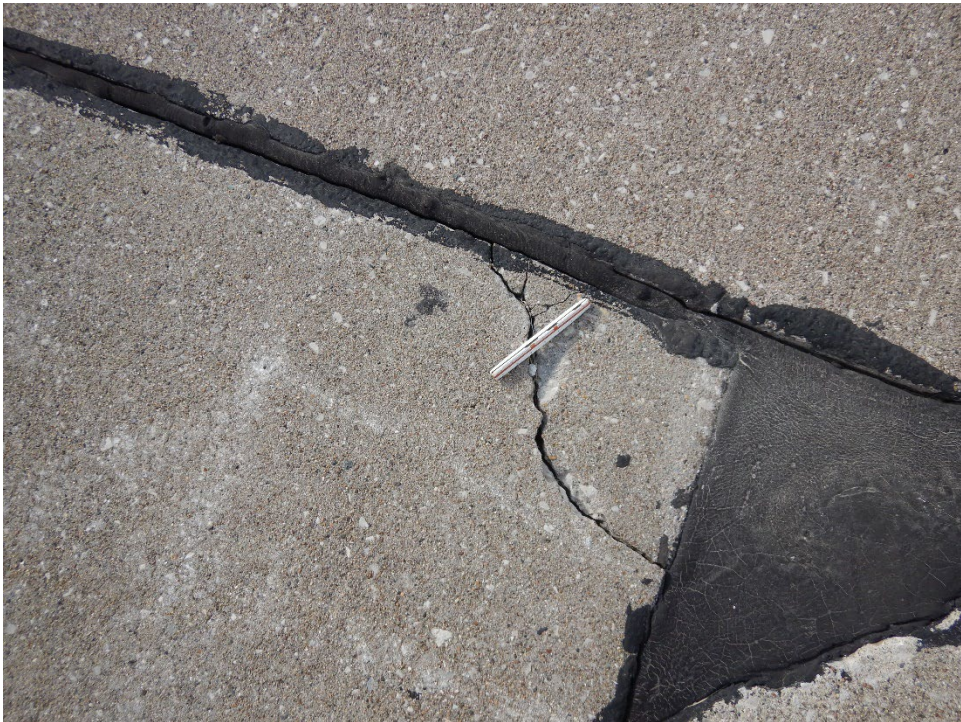
A01WA-04. Corner Spalling (Sample Unit No. 01).
