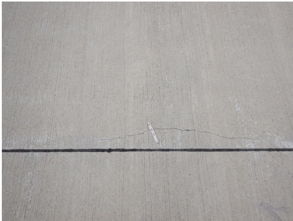
A01WA-08. Joint Spalling (Sample Unit No. 02).
