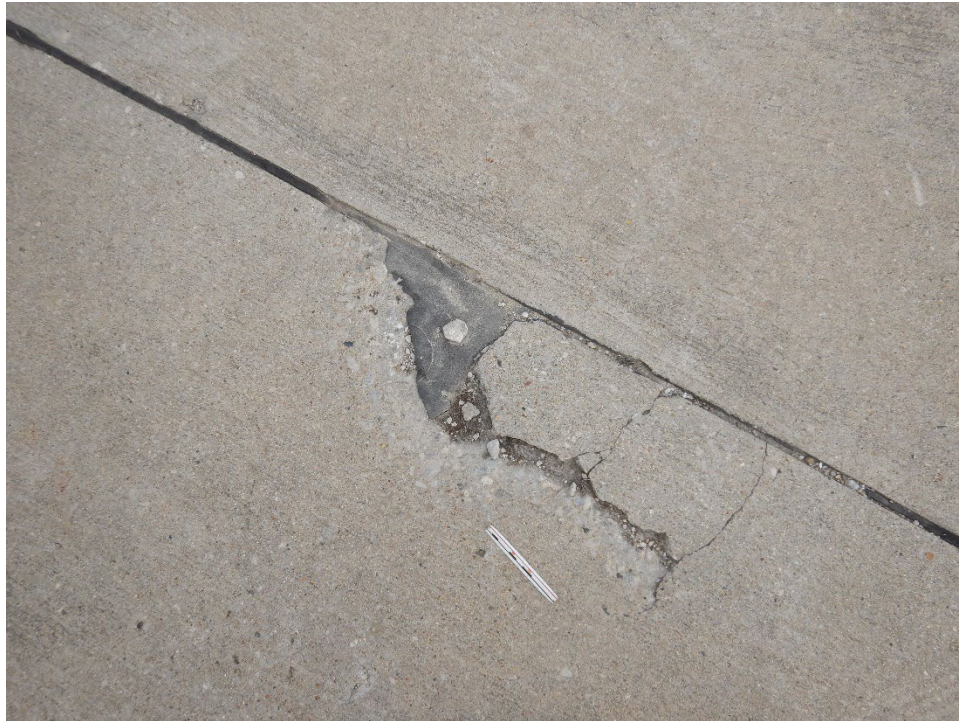
TH01WA-02. Joint Spalling (Sample Unit No. 01).
