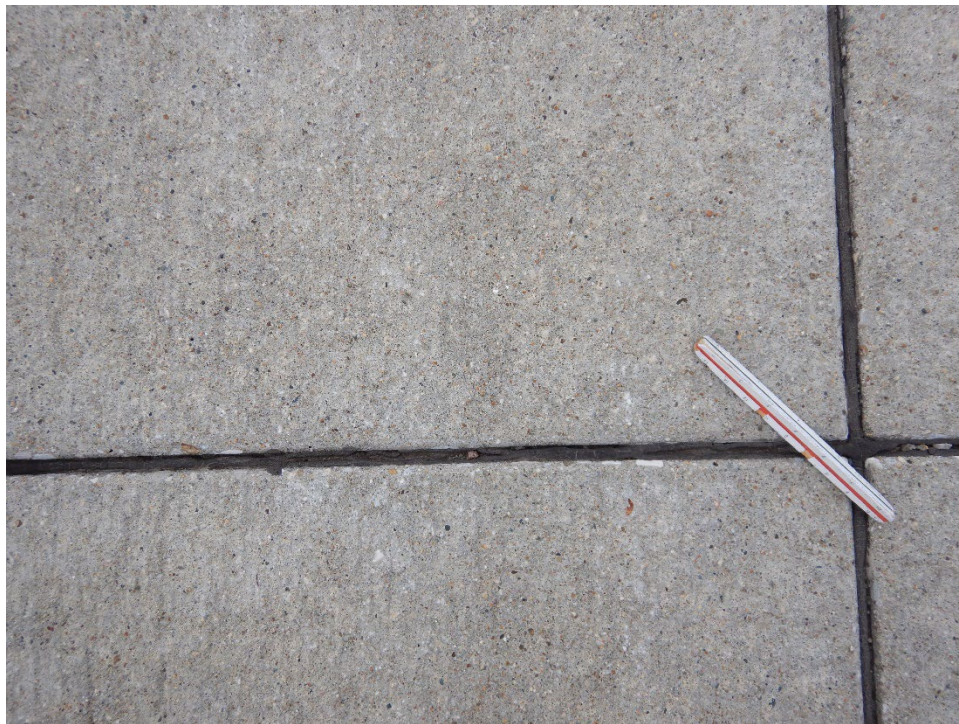
T01WA-02. Joint Seal Damage (Sample Unit No. 04).
