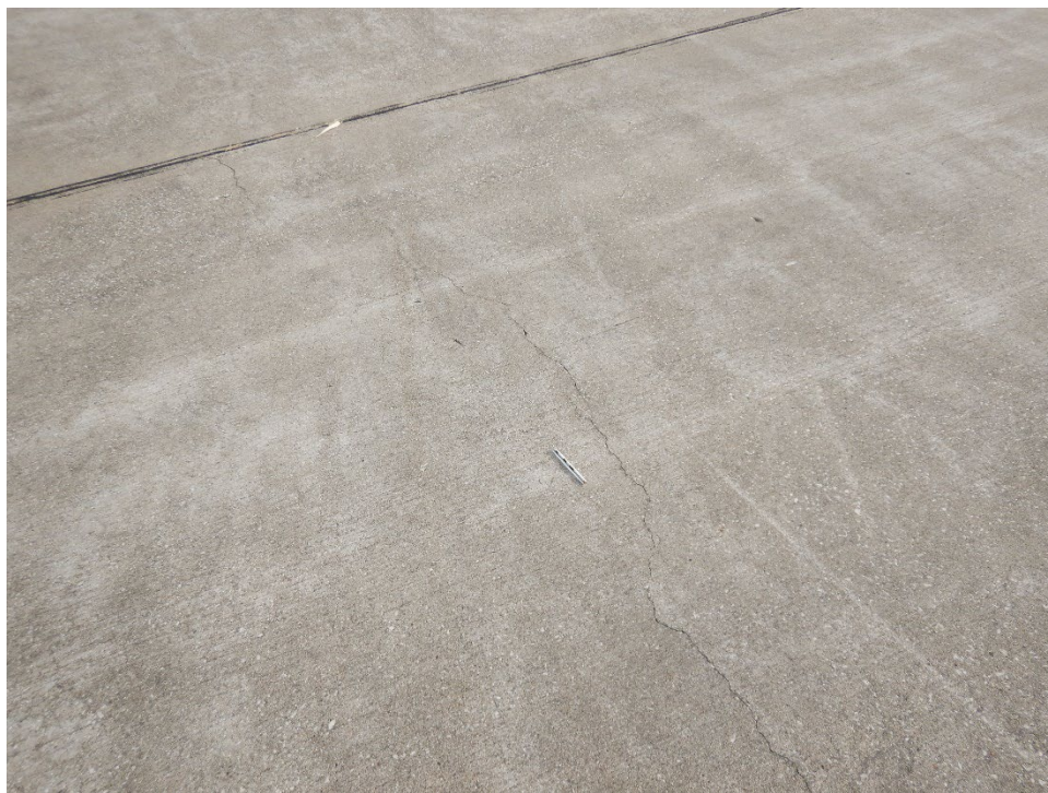
A01WA-03. LTD Cracking (Sample Unit No. 01).
