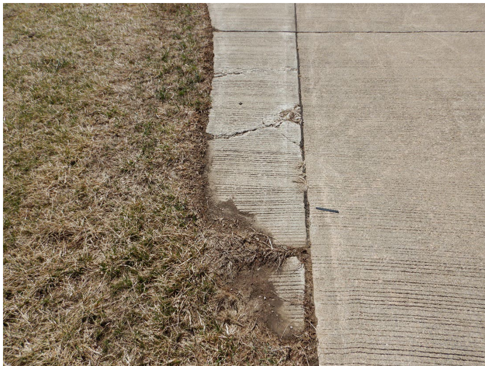
TCSL-01. Shattered Slab (Sample Unit No. 05).
