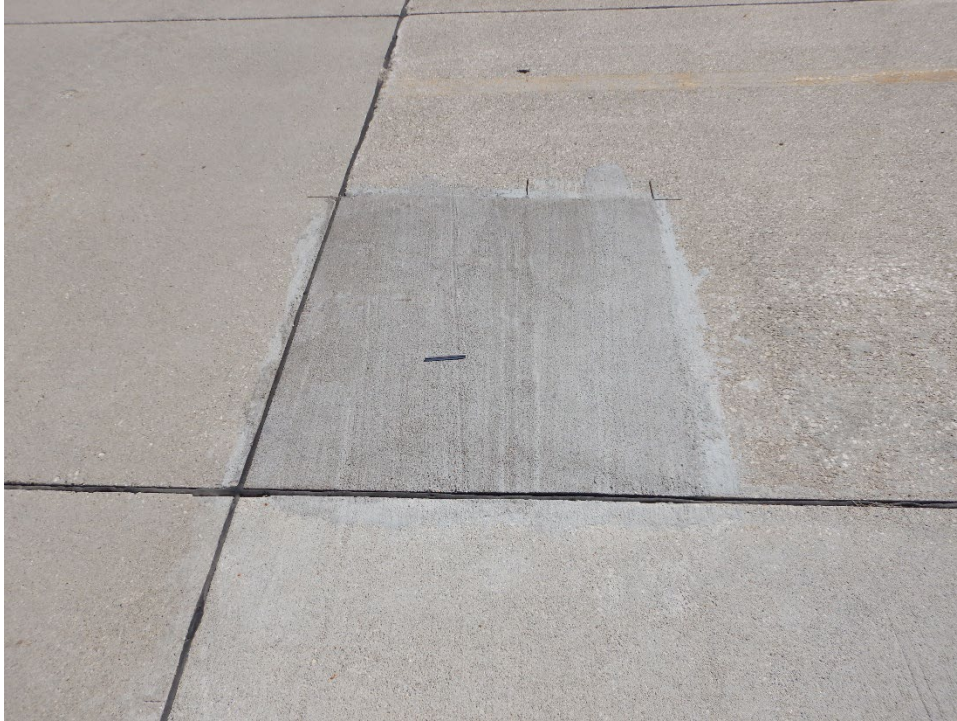
A01SL-02. Large Patching (Sample Unit No. 03).
