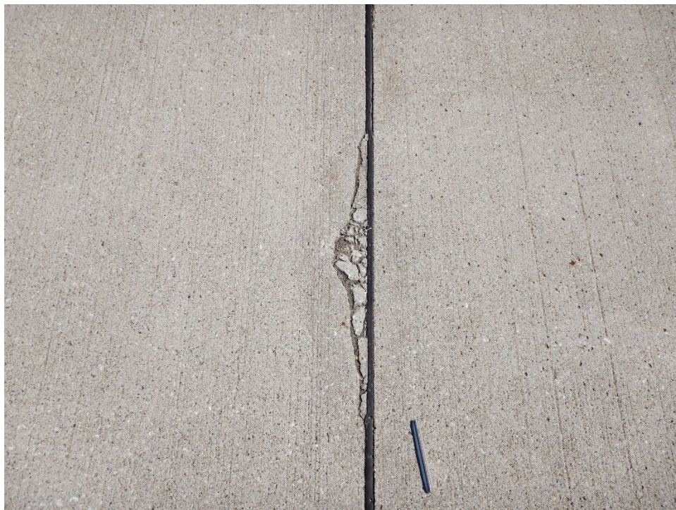
TA1SL-01. Joint Spalling (Sample Unit No. 02).
