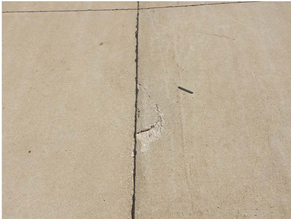
TH01SL-03. Joint Spalling (Sample Unit No. 01).
