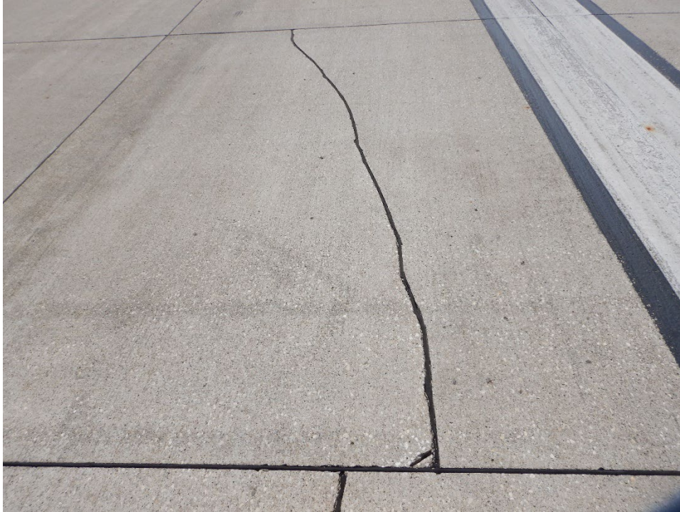
R17SL-02. LTD Cracking (Sample Unit No. 04).
