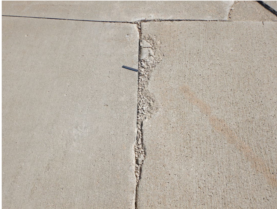
TH01SL-01. Joint Spalling (Sample Unit No. 04).
