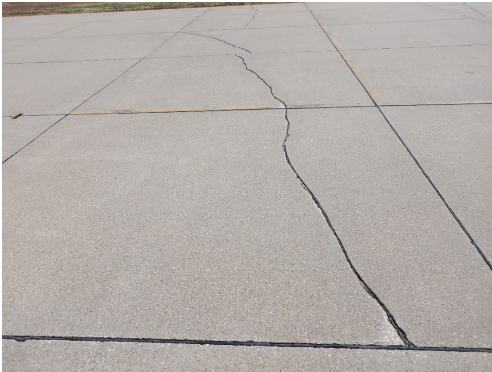
A01SL-01. LTD Cracking (Sample Unit No. 06).
