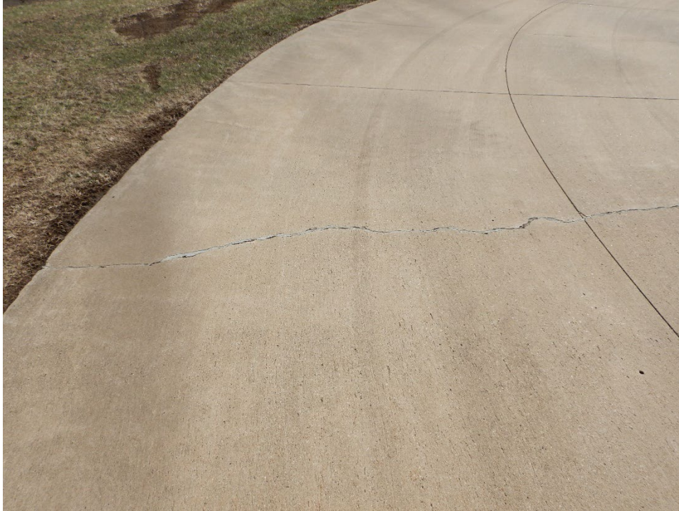
TH01SL-02. LTD Cracking (Sample Unit No. 02).
