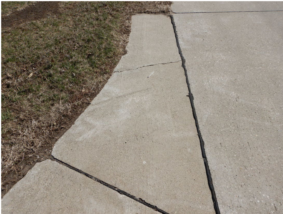
TH01SL-04. LTD Cracking (Sample Unit No. 01).
