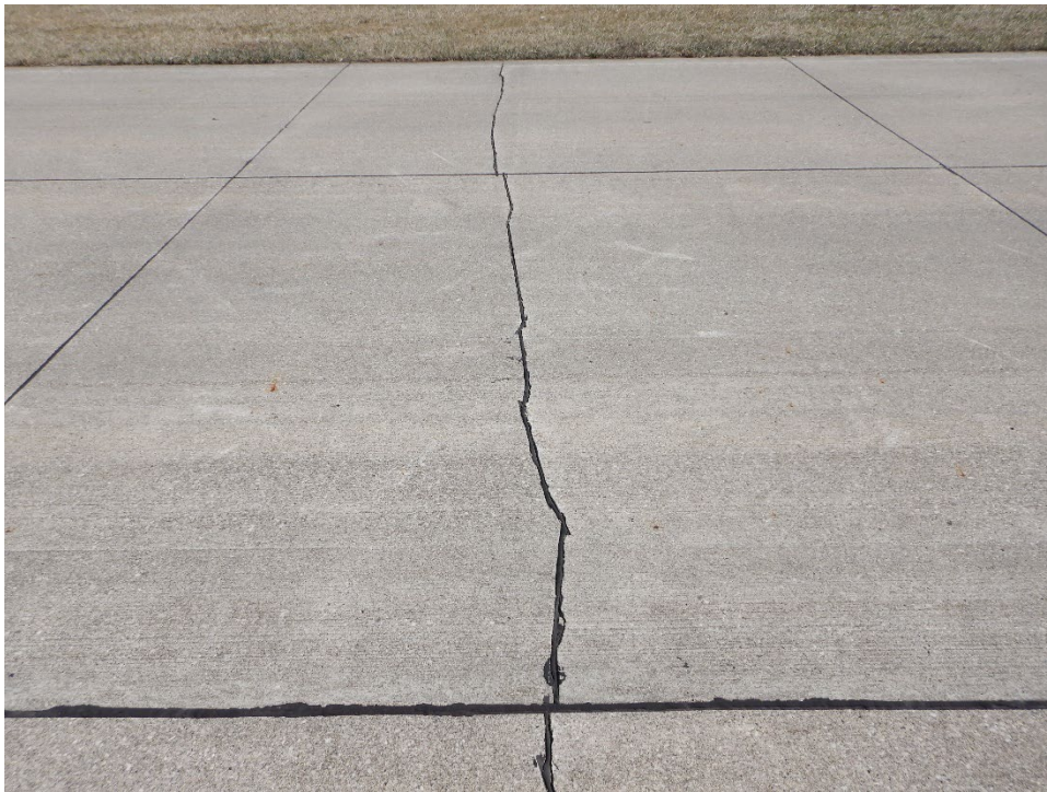
R17SL-01. LTD Cracking (Sample Unit No. 48).
