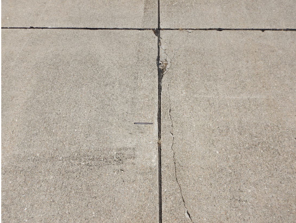
R13SL-01. Joint Spalling (Sample Unit No. 03).
