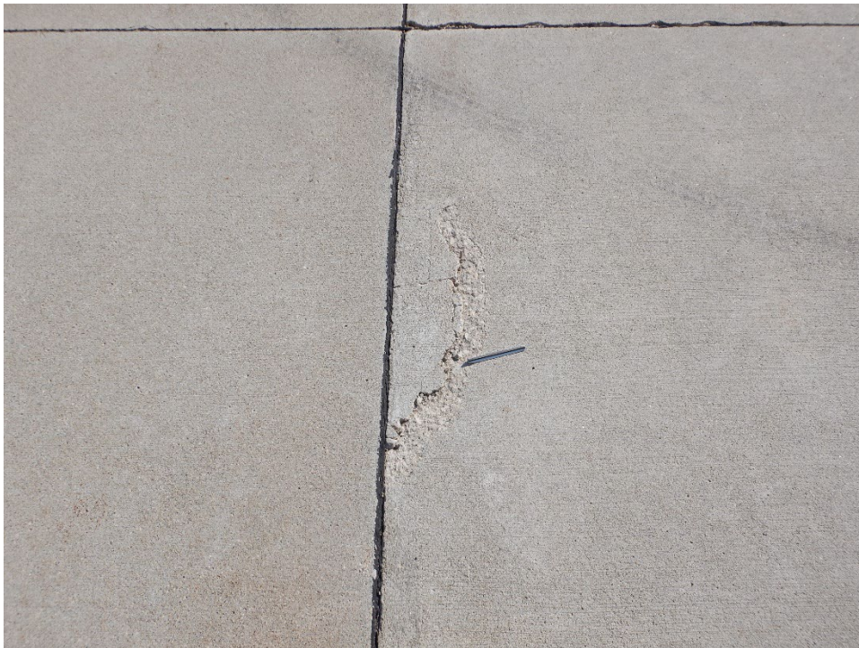
TH01SL-01. Joint Spalling (Sample Unit No. 01).
