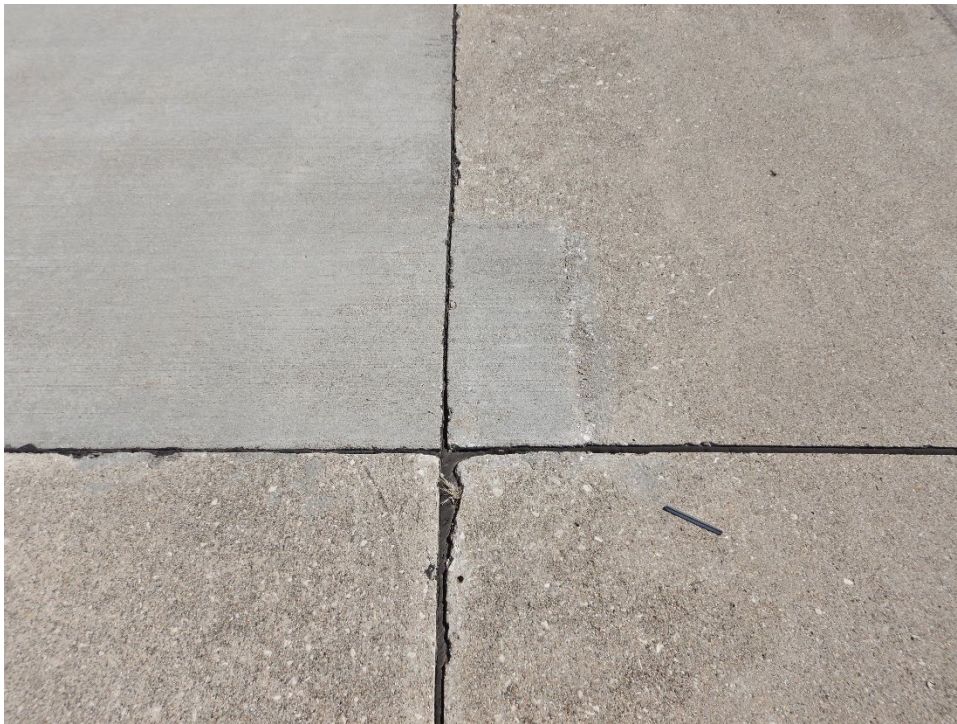
R13SL-01. Small Patching (Sample Unit No. 03).
