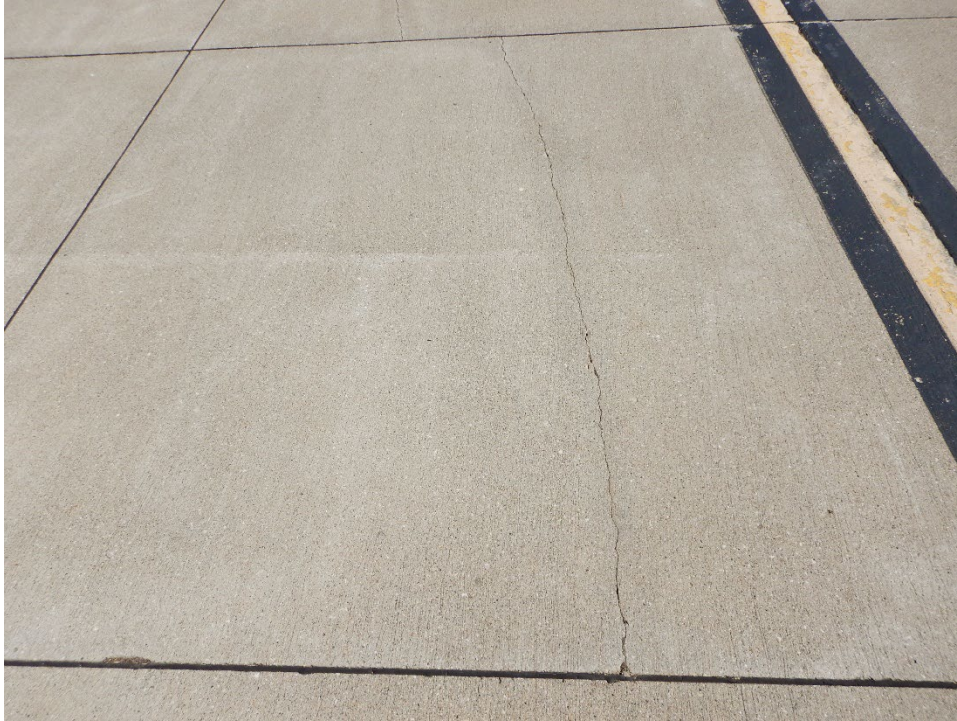
TA1SL-01. LTD Cracking (Sample Unit No. 04).
