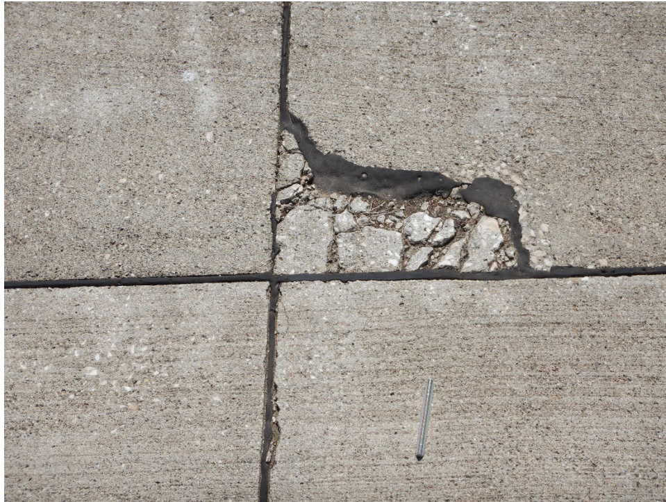
TA1SL-01. Corner Spalling (Sample Unit No. 04).
