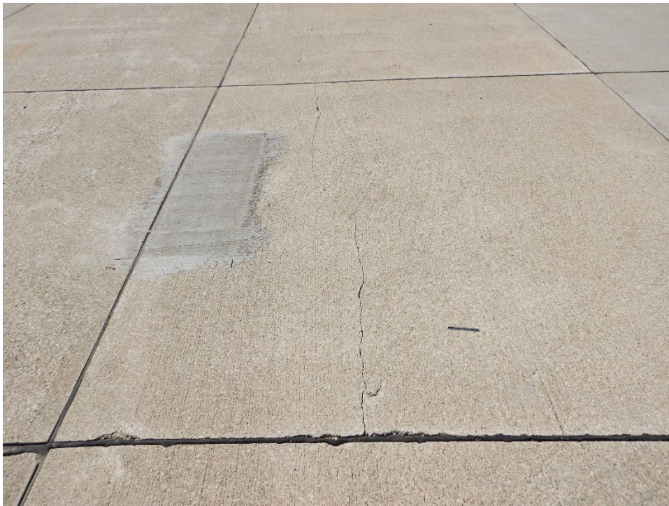
A01SL-02. LTD Cracking (Sample Unit No. 03).
