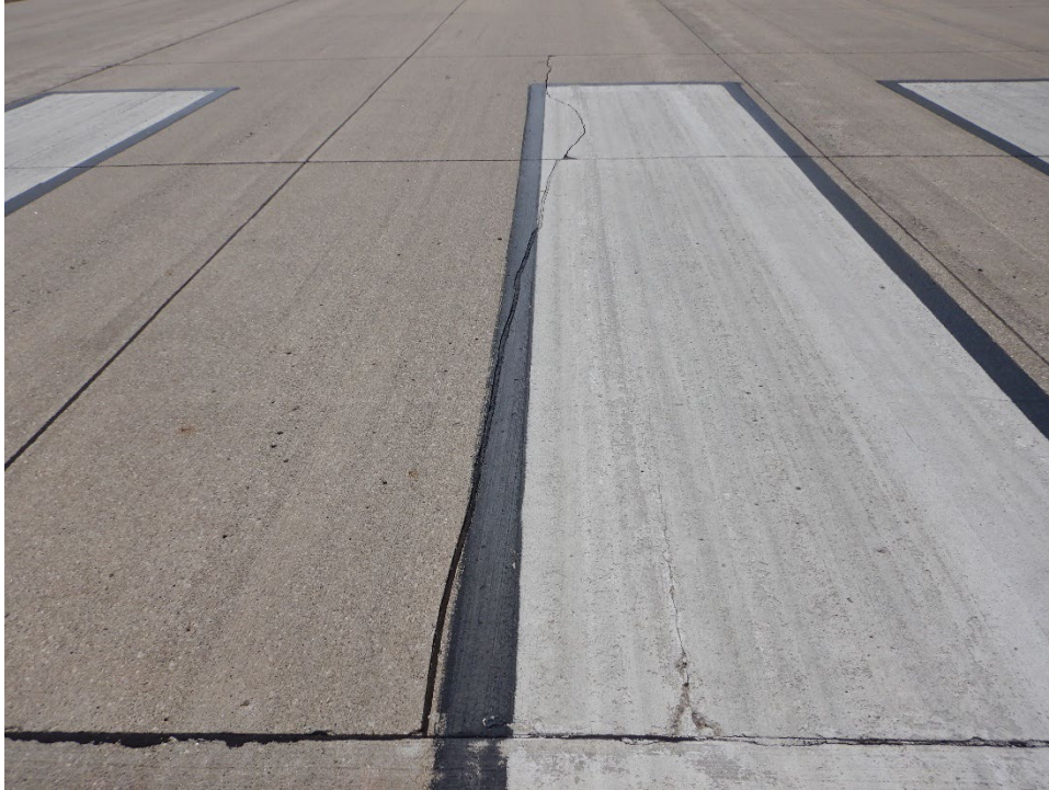
R17SL-01. LTD Cracking (Sample Unit No. 03).
