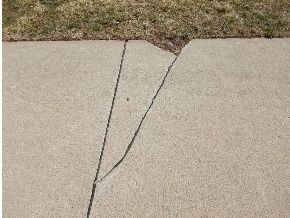
TCSL-01. LTD Cracking (Sample Unit No. 04).
