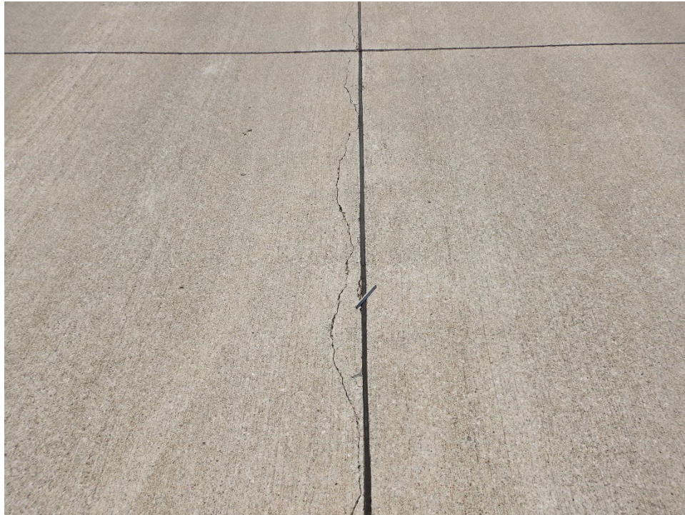
TCSL-02. Joint Spalling (Sample Unit No. 04).
