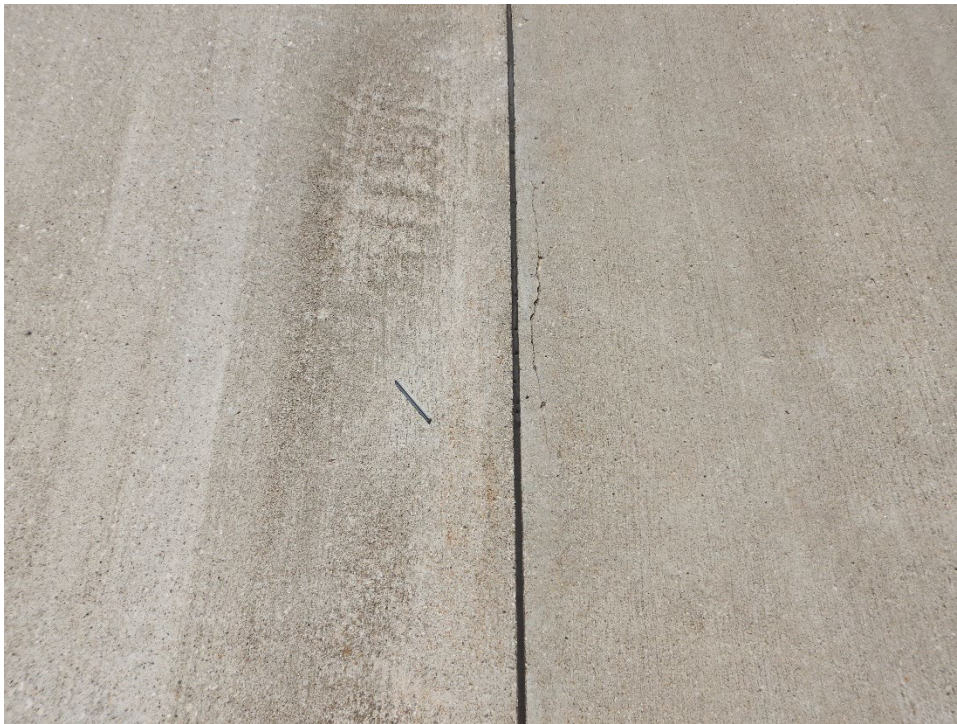
R17SL-02. Joint Spalling (Sample Unit No. 04).
