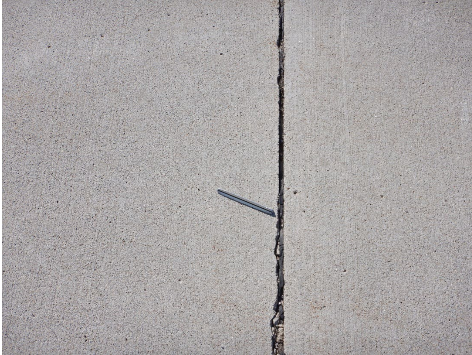
TH01SL-01. Joint Seal Damage (Sample Unit No. 01).
