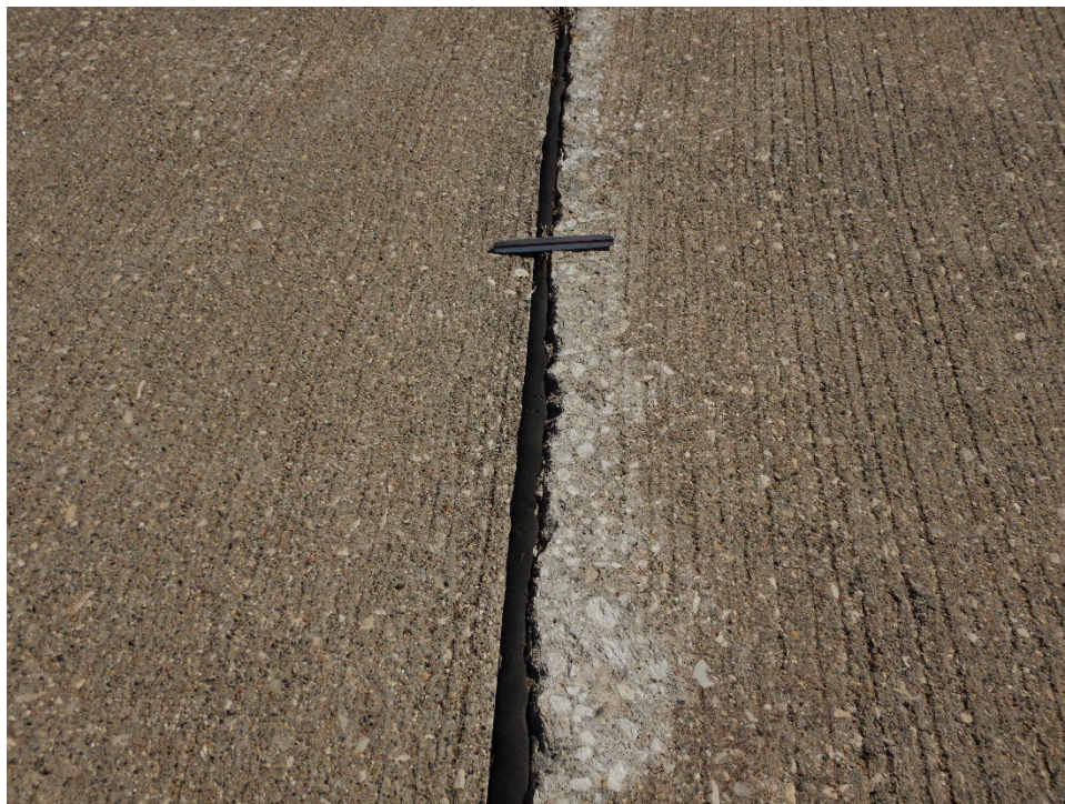
TCSL-01. Faulting (Sample Unit No. 02).
