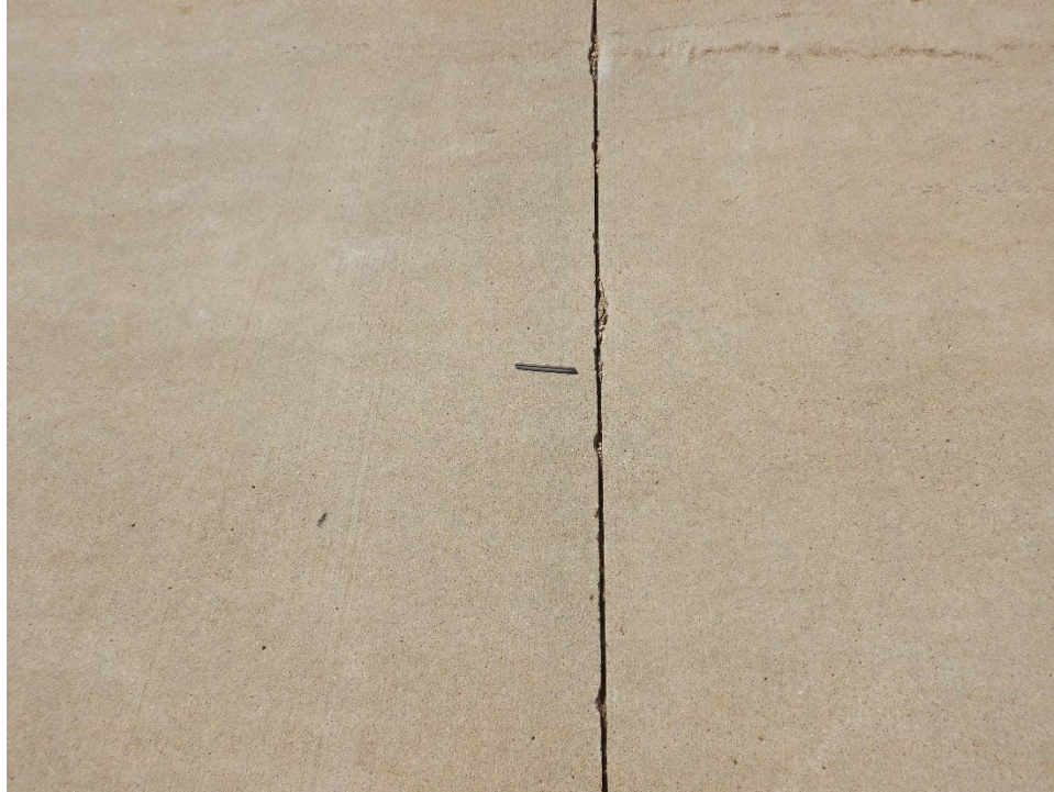
TH01SL-03. Joint Seal Damage (Sample Unit No. 01).
