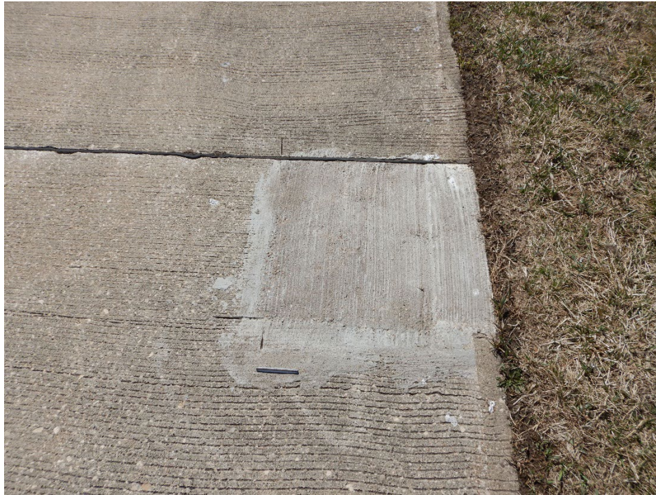
TCSL-01. Small Patching (Sample Unit No. 01).
