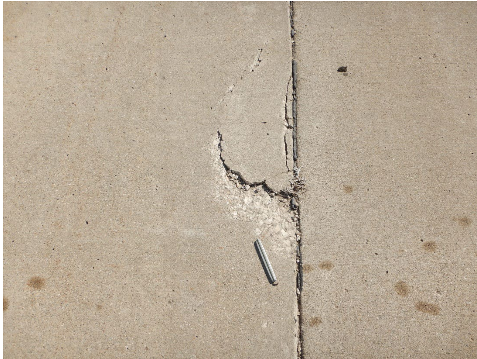
TH01SL-02. Joint Spalling (Sample Unit No. 05) (1).
