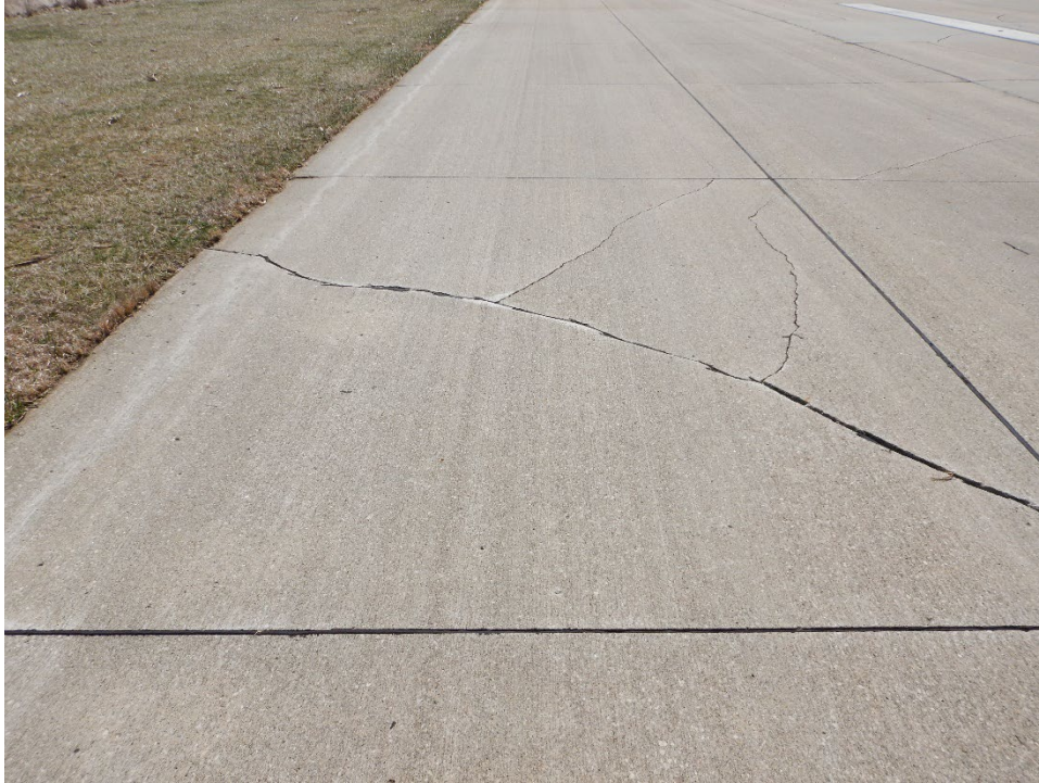
R17SL-01. Shattered Slab (Sample Unit No. 38).
