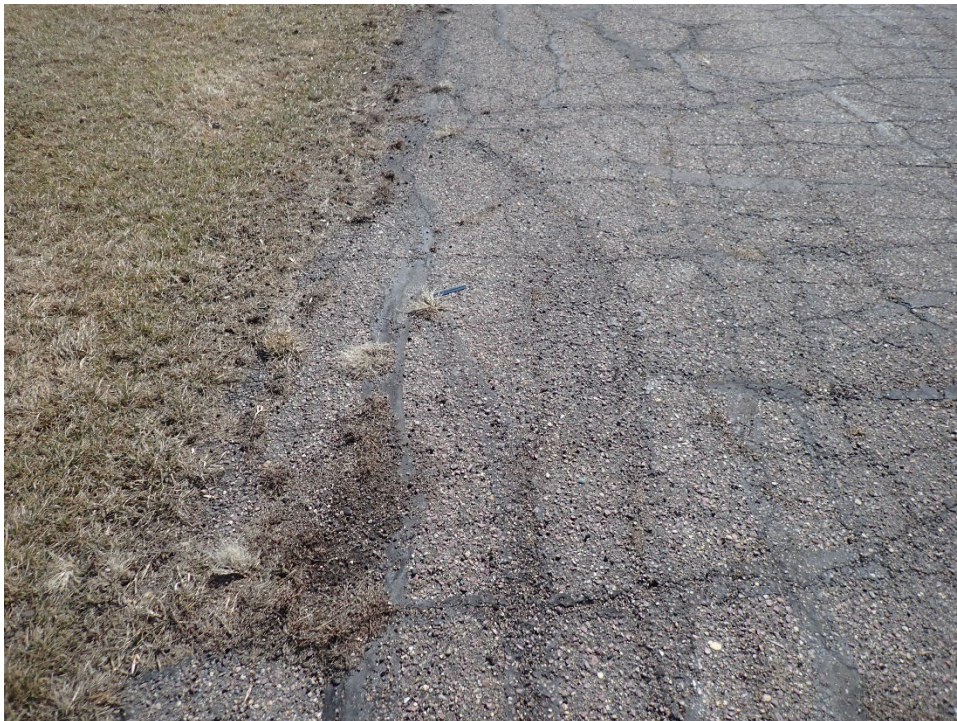
A015I-01. Alligator Cracking (Sample Unit No. 02).
