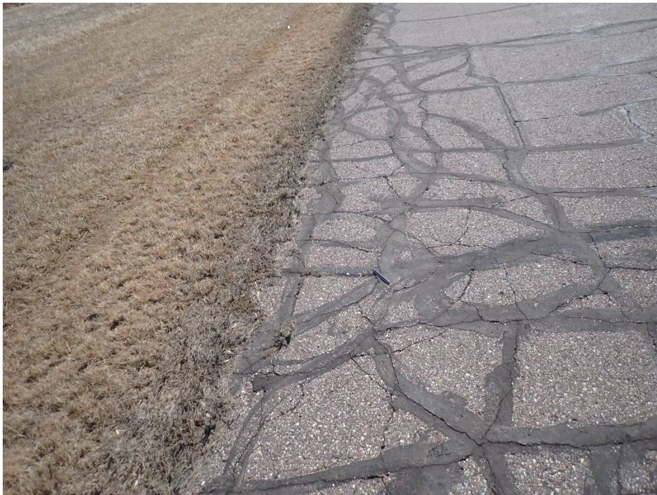
R165I-01. Alligator Cracking (Sample Unit No. 02).
