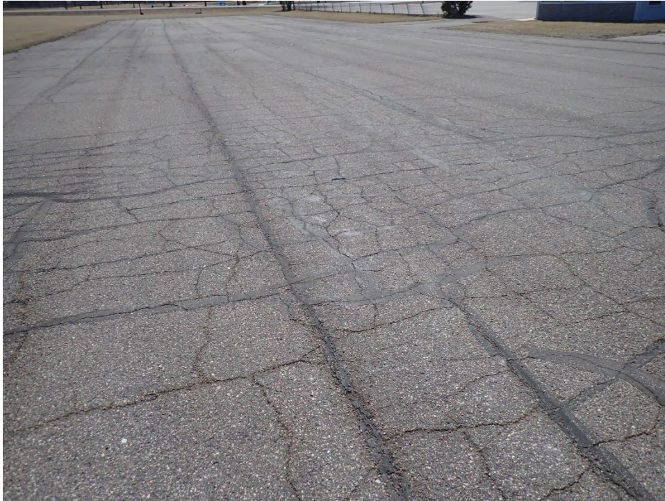
A015I-01. Alligator Cracking (Sample Unit No. 04).
