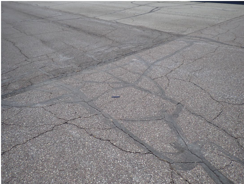
T015I-01. Alligator Cracking (Sample Unit No. 02).
