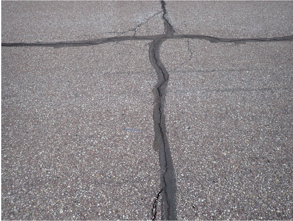
R165I-01. L&T Cracking (Sample Unit No. 07).
