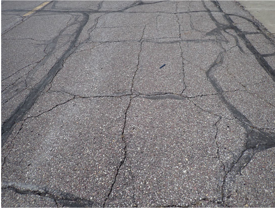
T015I-01. Block Cracking (Sample Unit No. 02).
