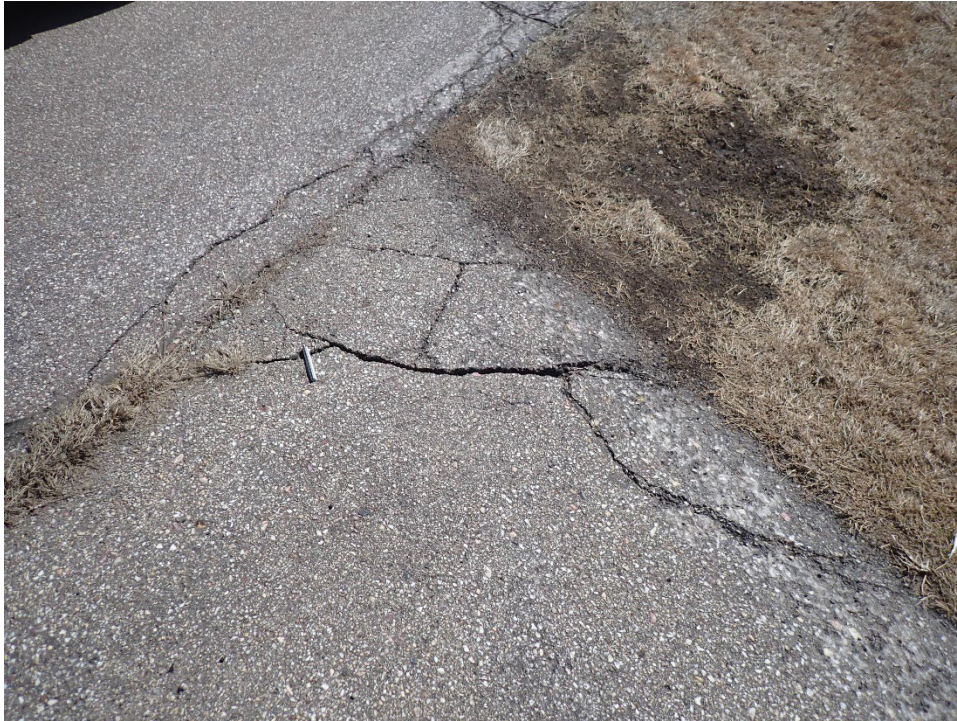
T025I-01. Alligator Cracking (Sample Unit No. 01).
