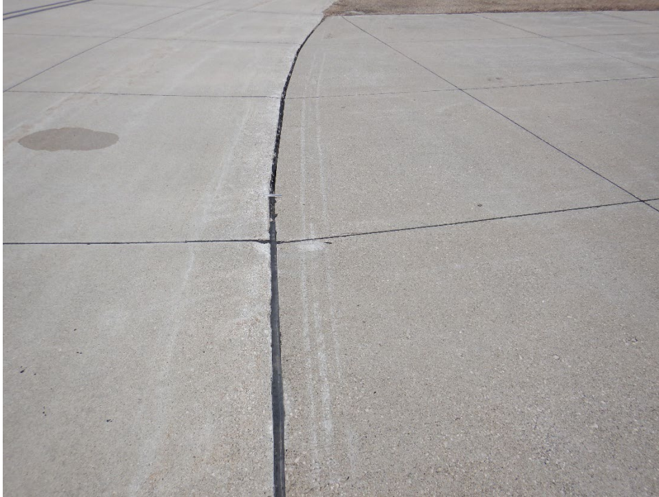
TB1SP-01. Faulting (Additional Sample Unit No. 01).
