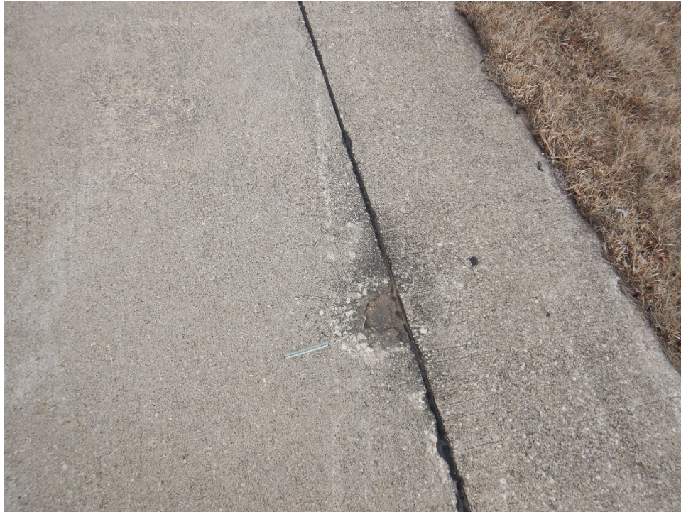
TC2SP-01. Joint Spalling (Sample Unit No. 03).
