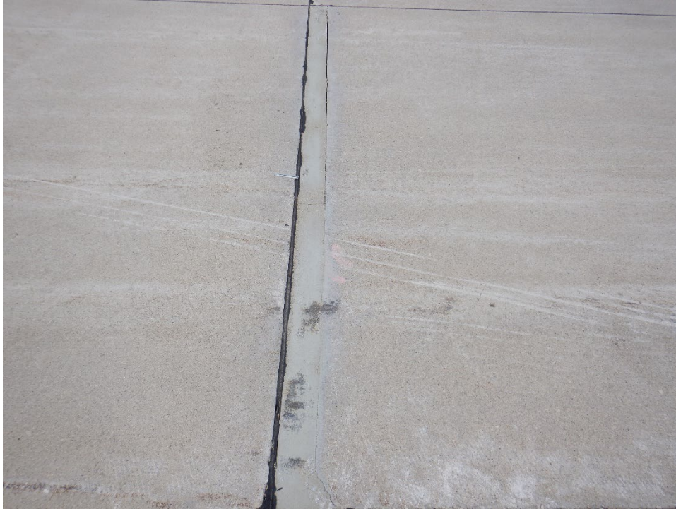
TESP-01. Large Patching (Sample Unit No. 01).
