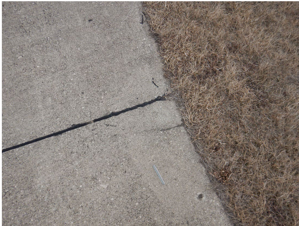
TC1SP-01. Shrinkage Cracking (Sample Unit No. 02).
