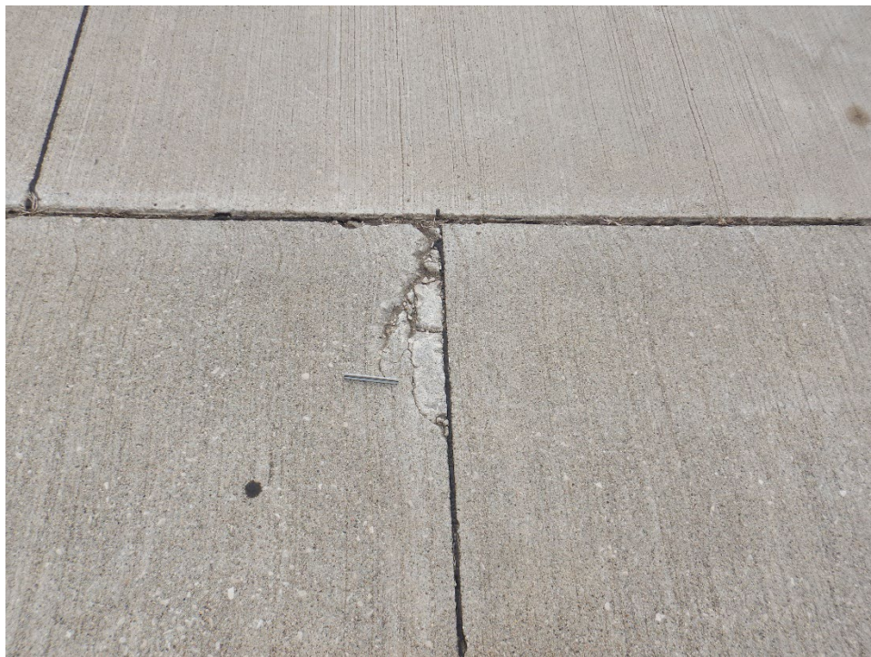
A01SP-02. Joint Spalling (Sample Unit No. 18).
