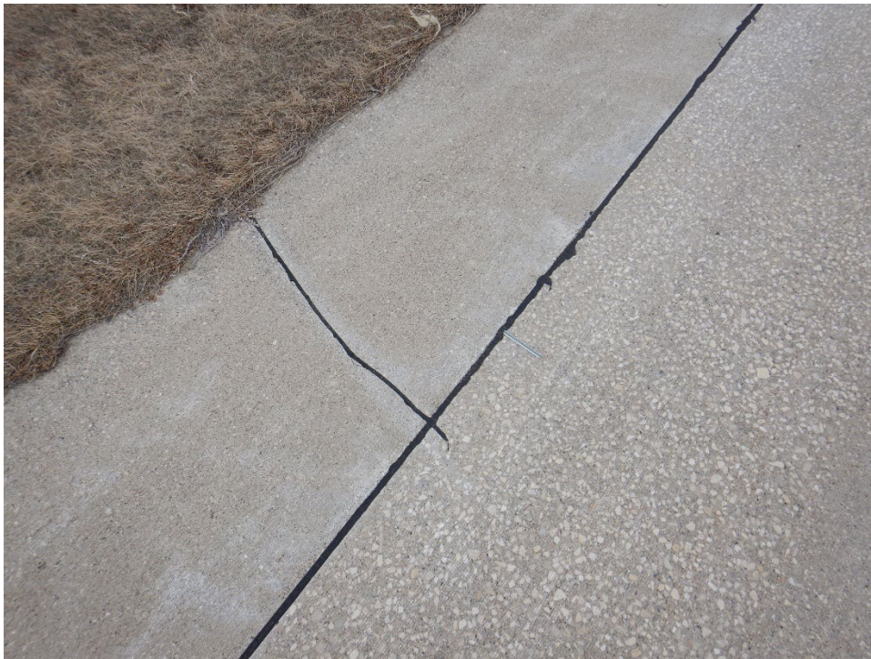
TESP-01. LTD Cracking (Sample Unit No. 15).
