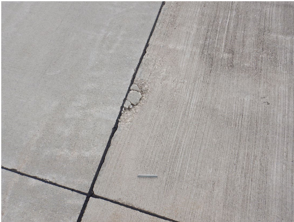
A01SP-03. Joint Spalling (Sample Unit No. 05).
