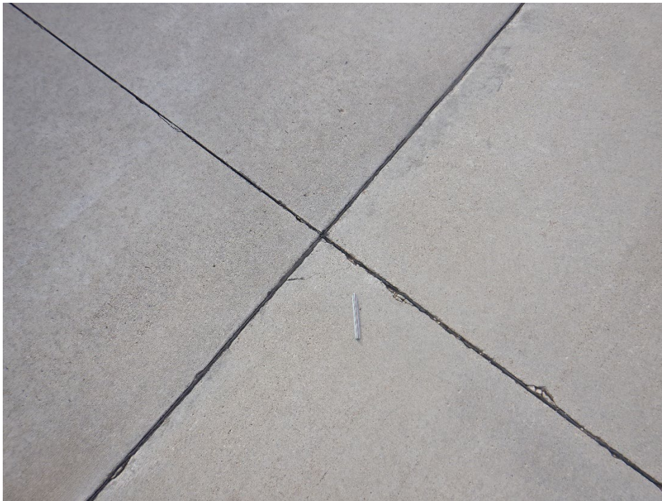
TH01SP-02. Corner Spalling (Sample Unit No. 01).
