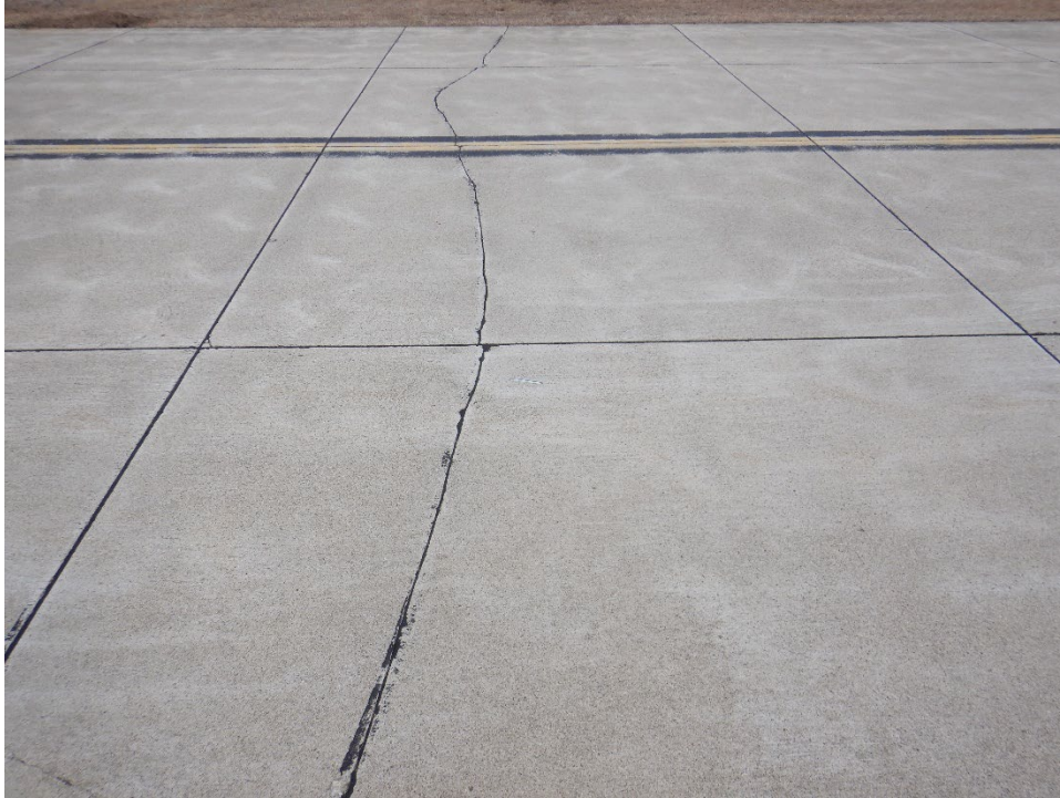
TCSP-02. LTD Cracking (Sample Unit No. 05).
