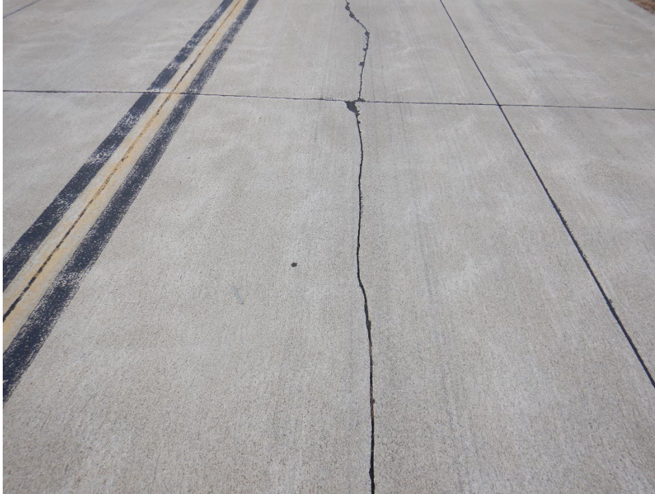
TCSP-01. LTD Cracking (Sample Unit No. 04).
