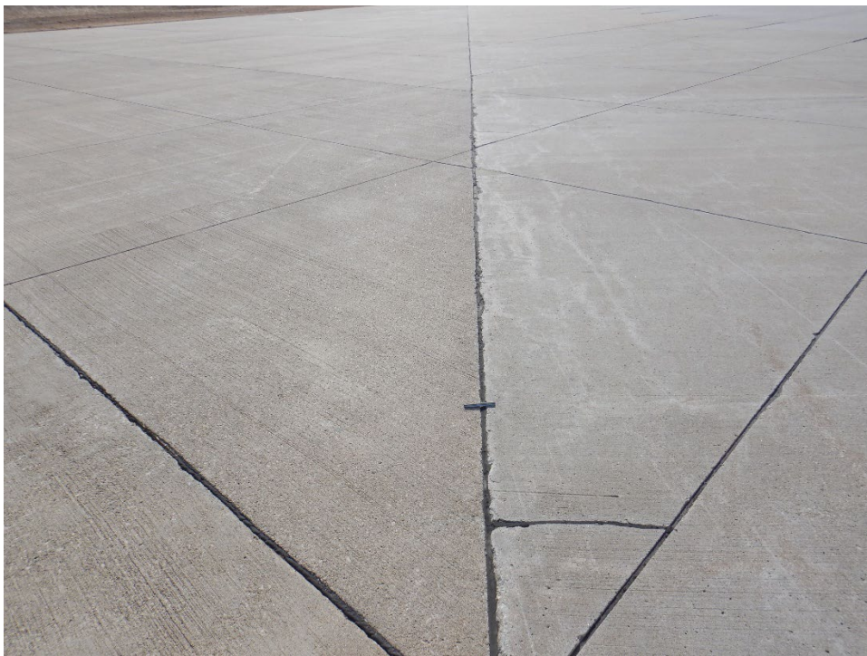
A01SP-03. Faulting (Sample Unit No. 11).
