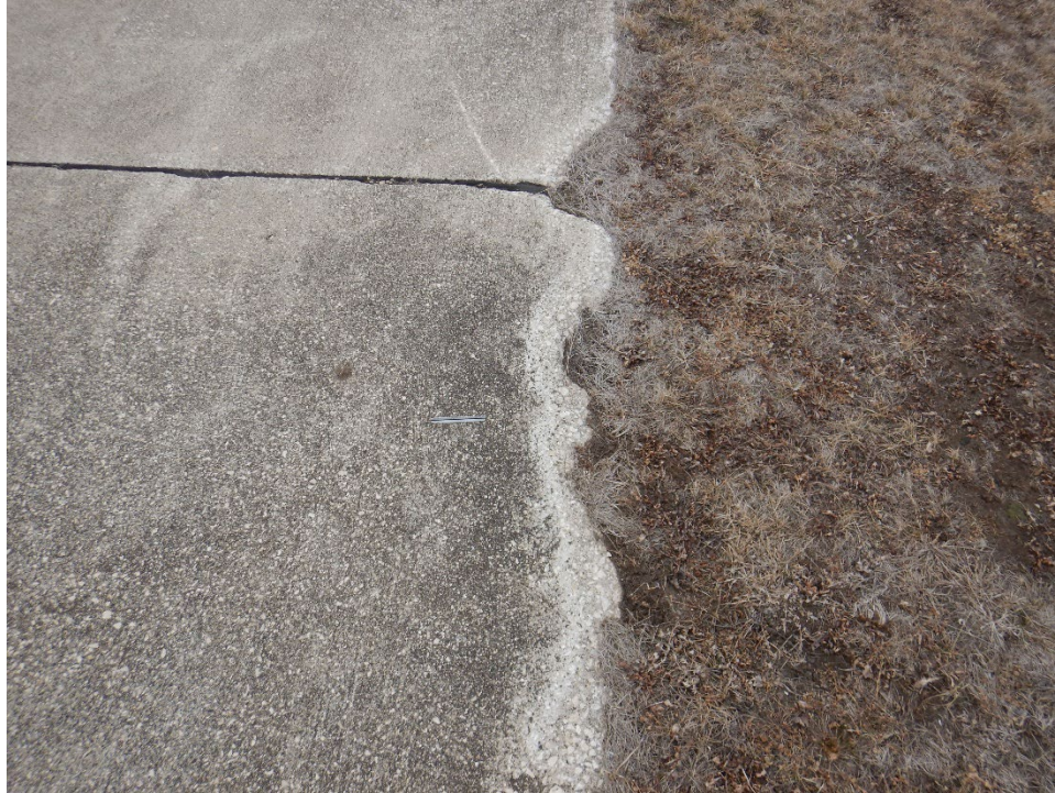
TC1SP-01. Joint Spalling (Additional Sample Unit No. 01).
