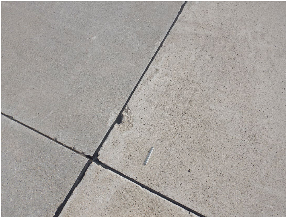
TASP-01. Joint Spalling (Sample Unit No. 02).
