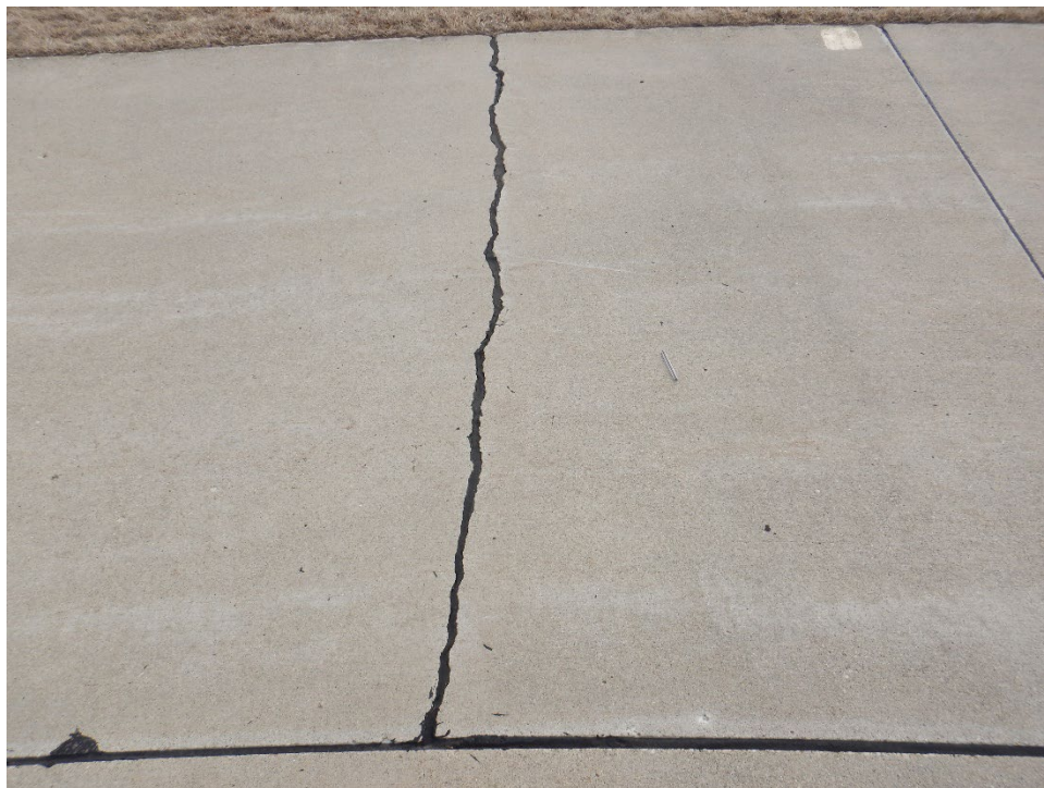
TDSP-01. LTD Cracking (Sample Unit No. 20).
