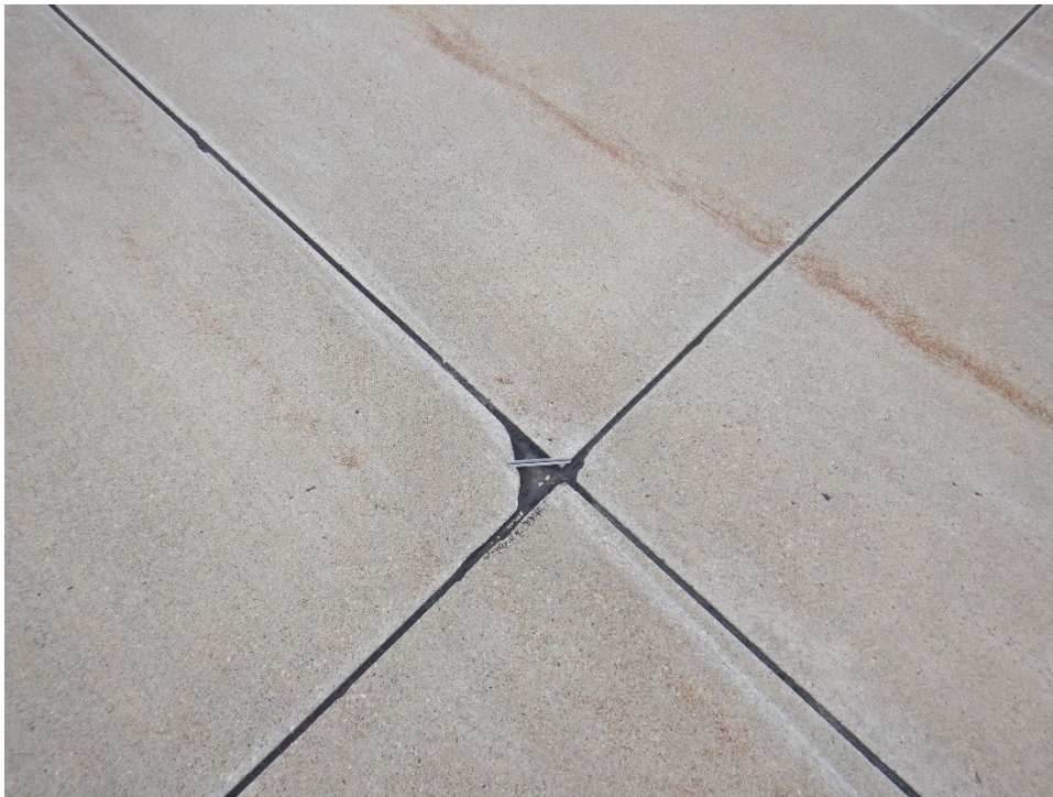
TBSP-01. Corner Spalling (Sample Unit No. 26).
