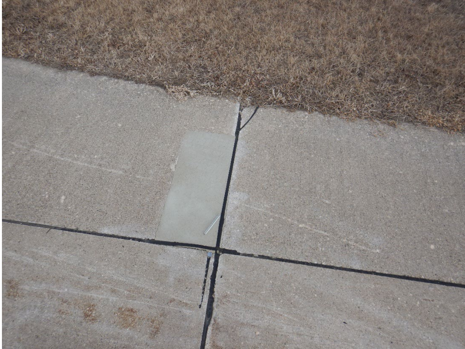
TASP-02. Small Patching (Sample Unit No. 13).
