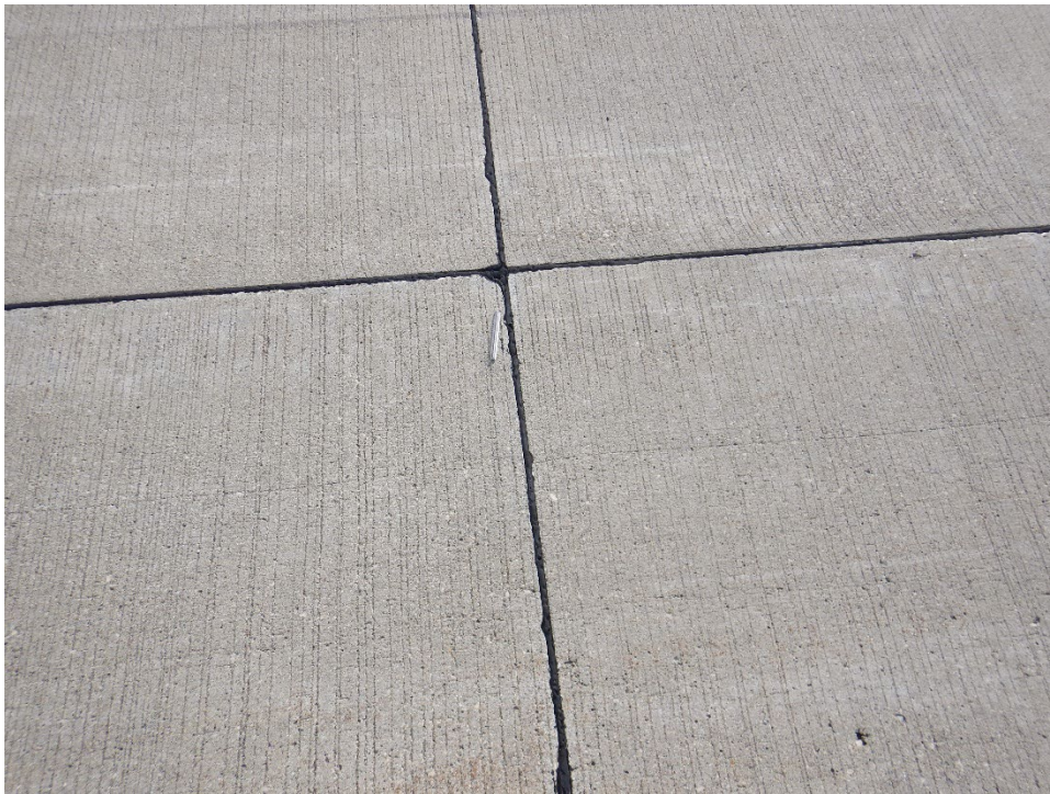
R18SP-01. Joint Seal Damage (Sample Unit No. 23).
