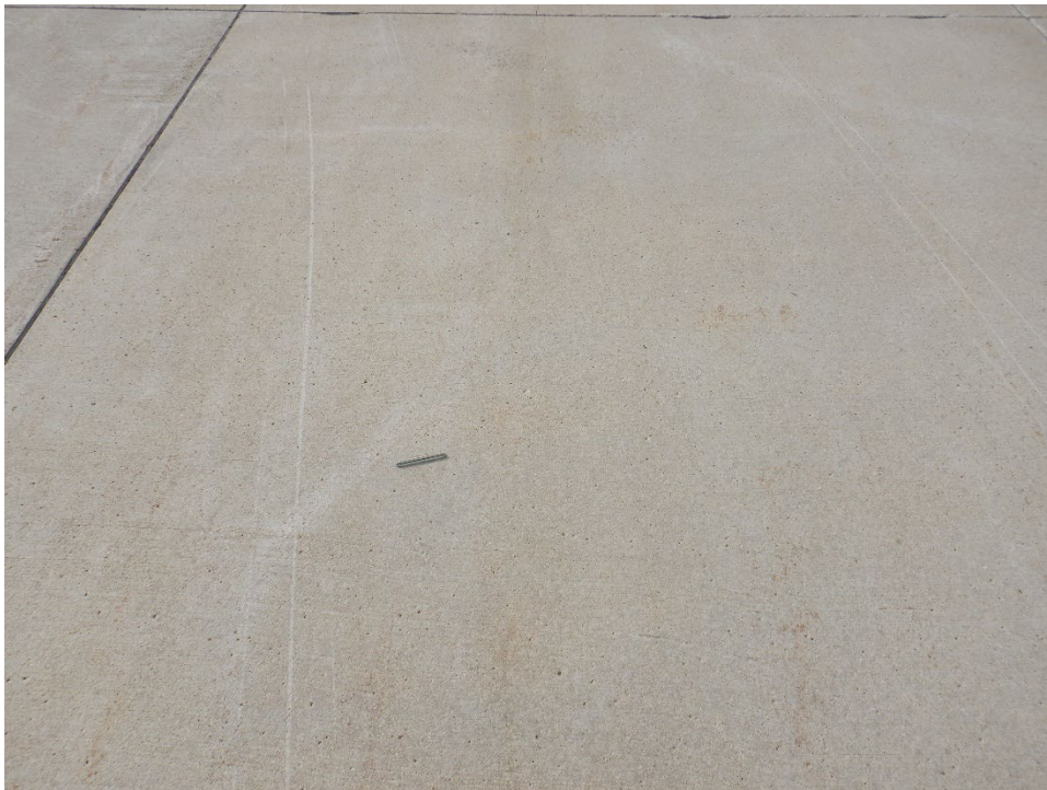
A01SP-02. Shrinkage Cracking (Sample Unit No. 14).
