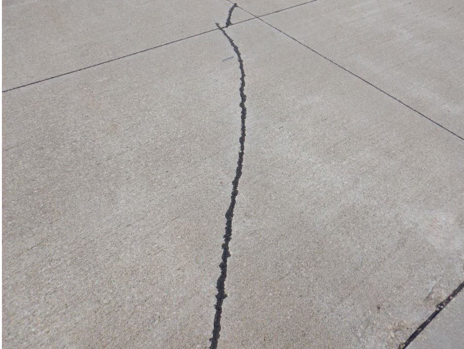
A01SP-02. LTD Cracking (Sample Unit No. 18).
