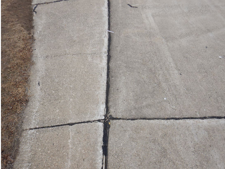
TCSP-03. Faulting (Additional Sample Unit No. 01).
