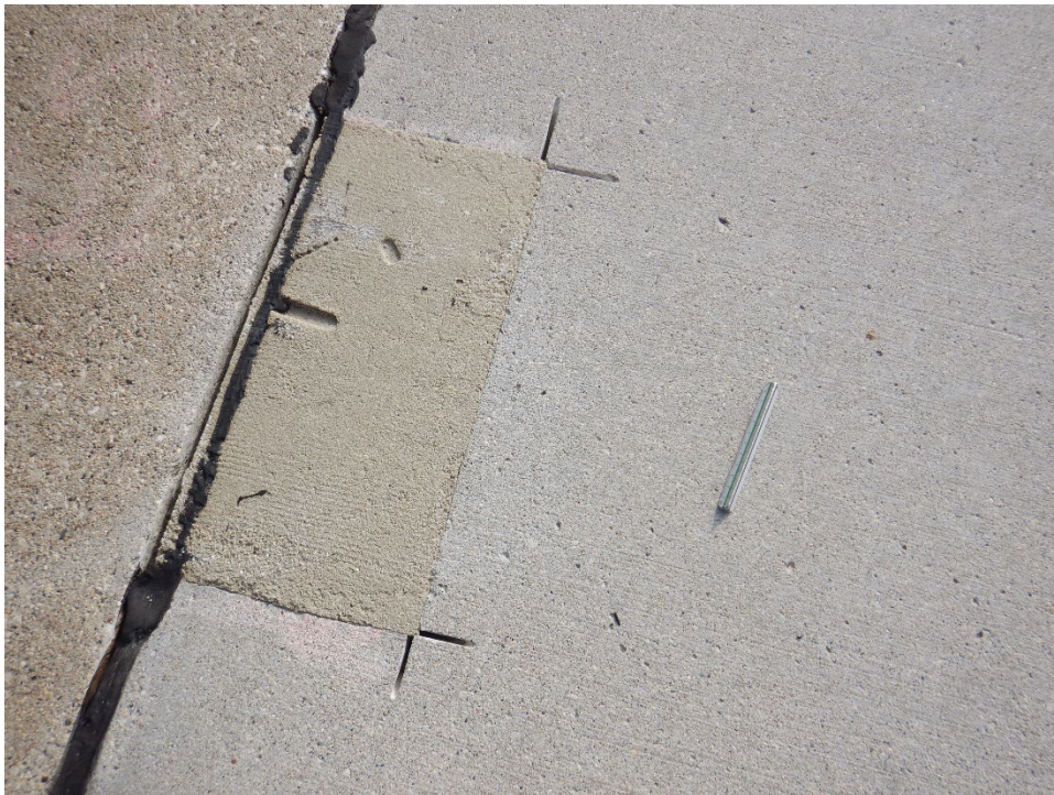
TH01SP-01. Small Patching (Sample Unit No. 01).
