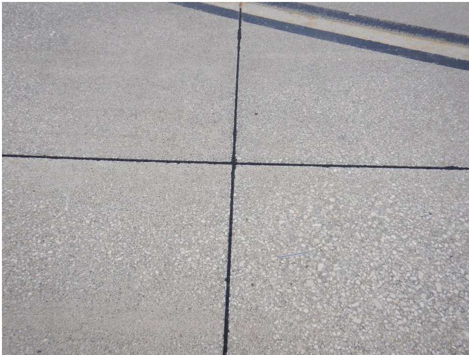
TC1SP-01. Joint Seal Damage (Sample Unit No. 02).
