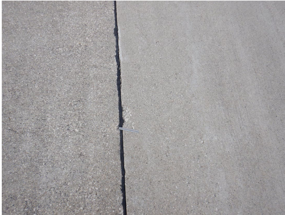
TCSP-03. Joint Seal Damage (Sample Unit No. 19) (2).
