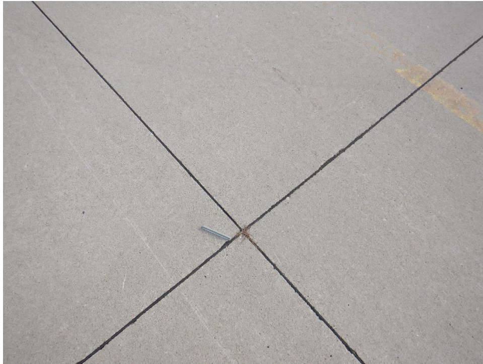
TH01SP-02. Joint Seal Damage (Sample Unit No. 01).
