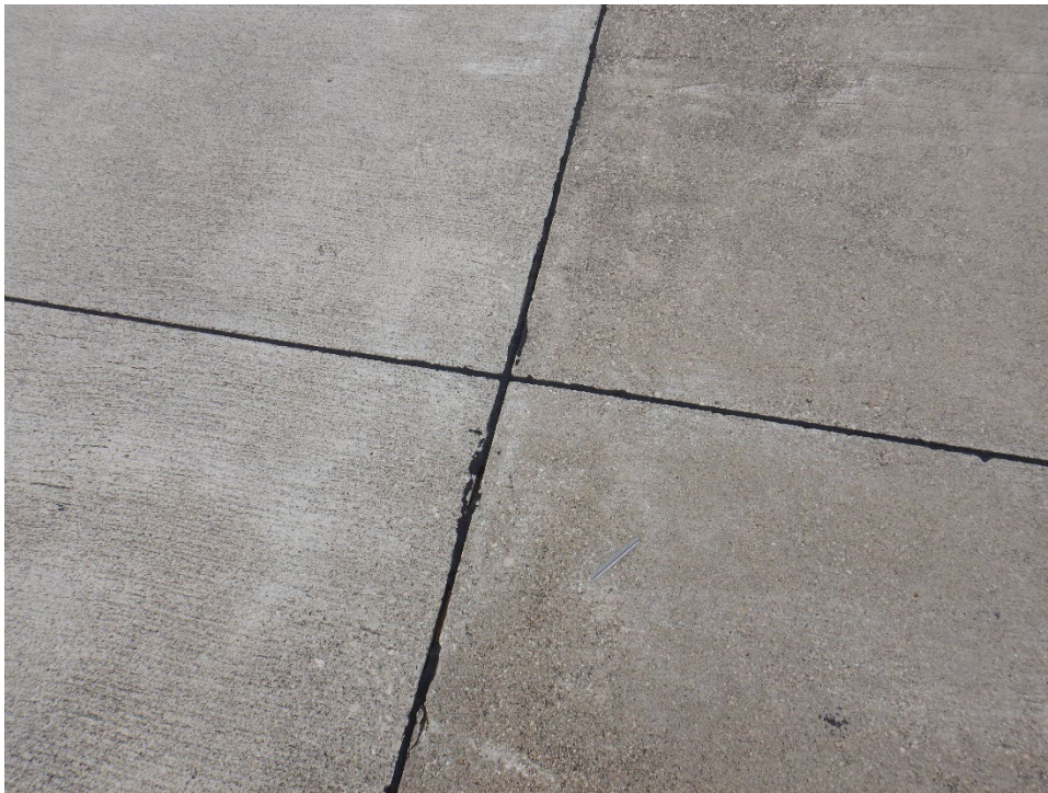
TC2SP-01. Joint Seal Damage (Sample Unit No. 03).
