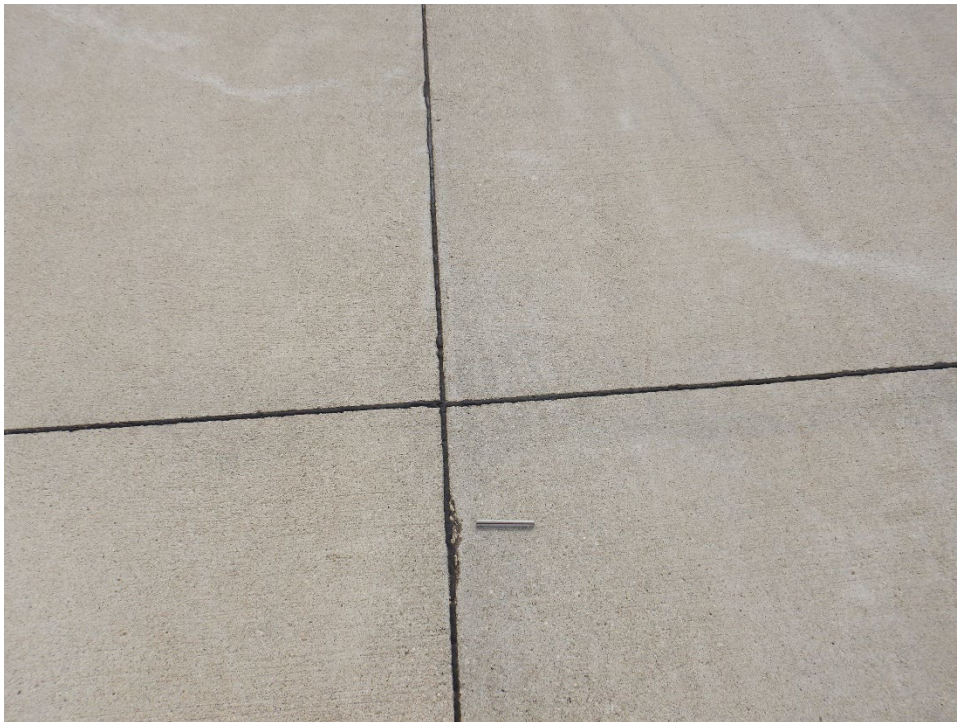
A01SP-07. Joint Seal Damage (Sample Unit No. 02).
