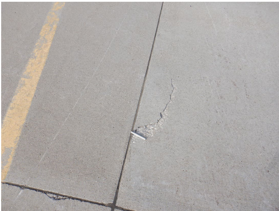
A01SP-06. Joint Spalling (Sample Unit No. 02).
