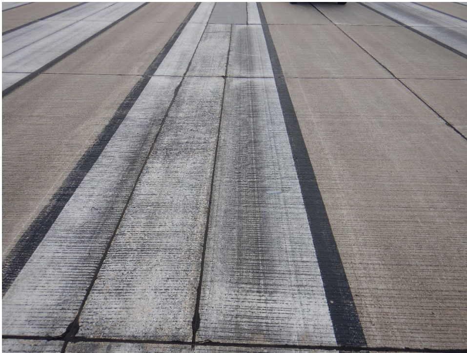
R12SP-01. Large Patching (Sample Unit No. 06).
