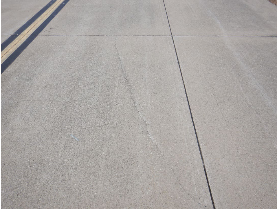
TB1SP-01. LTD Cracking (Sample Unit No. 03).
