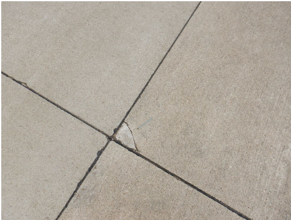
TH01SP-04. Corner Spalling (Sample Unit No. 08).
