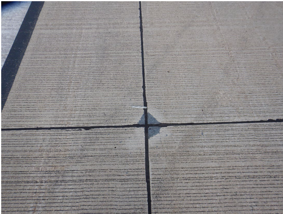
R12SP-01. Small Patching (Sample Unit No. 43).
