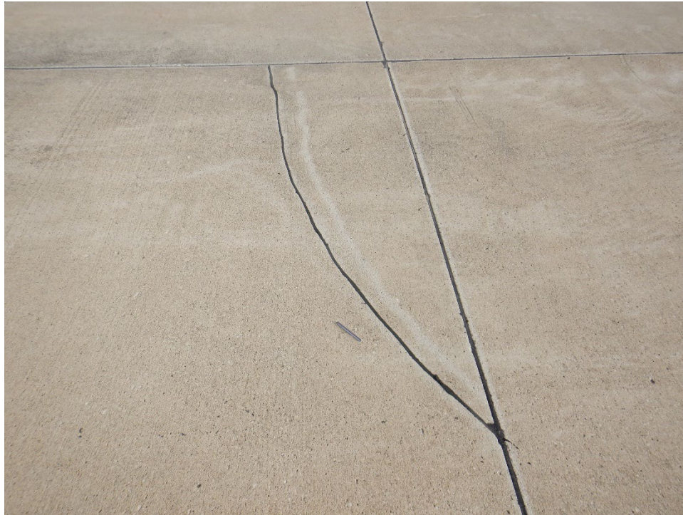
A01SP-05. LTD Cracking (Sample Unit No. 04).
