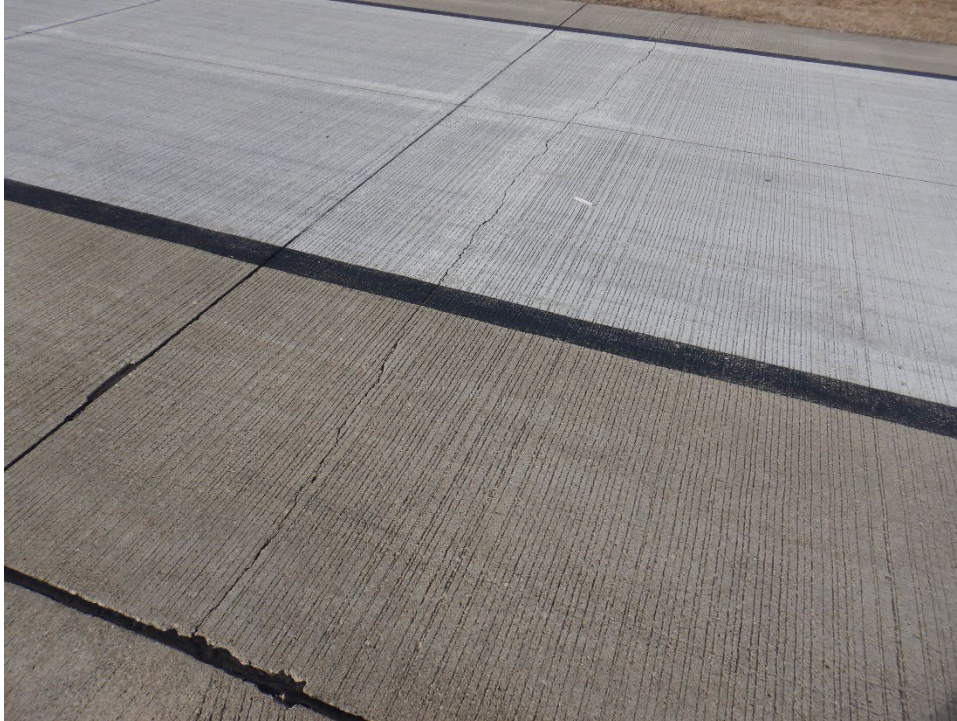
R18SP-01. LTD Cracking (Additional Sample Unit No. 22).
