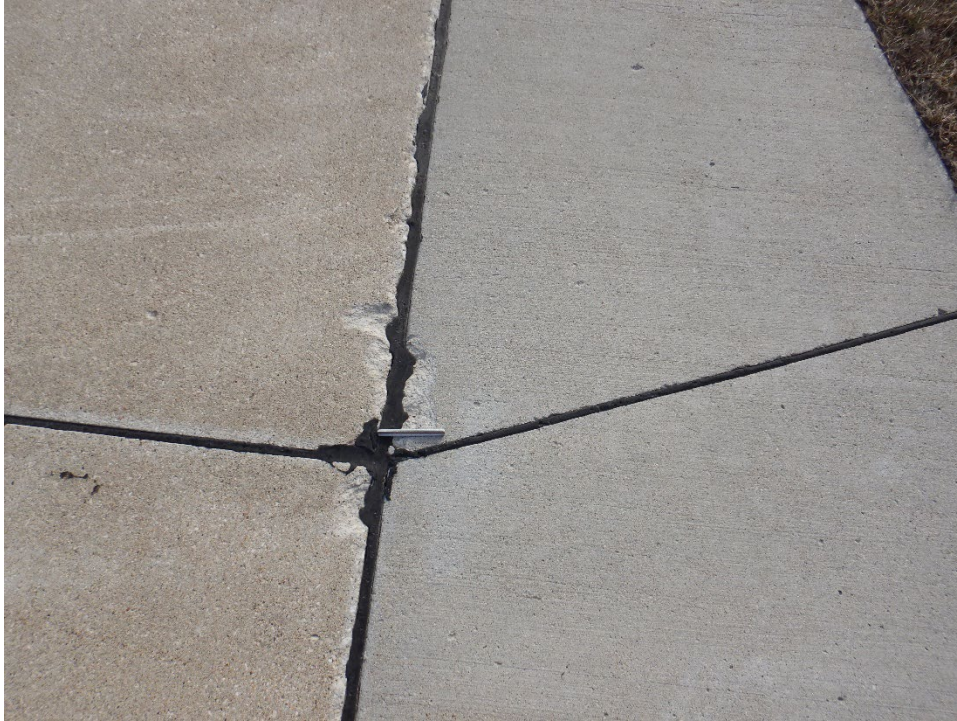
TH01SP-01. Joint Spalling (Sample Unit No. 01).
