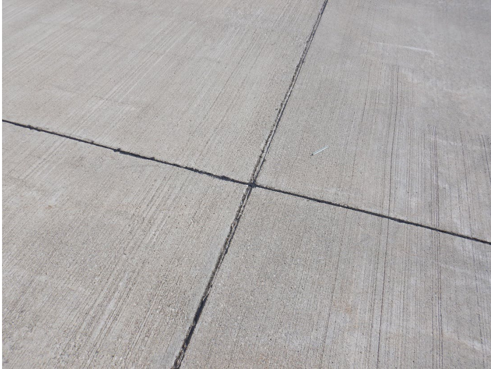
A01SP-03. Joint Seal Damage (Sample Unit No. 18).
