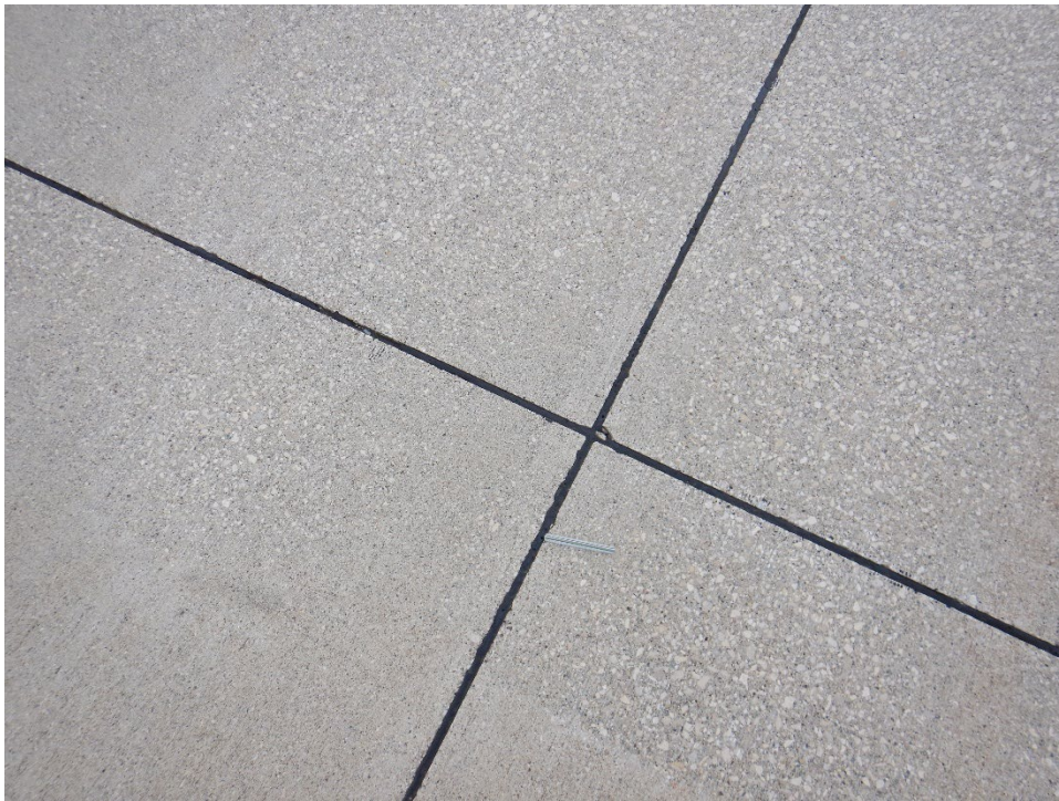
TCSP-03. Joint Seal Damage (Sample Unit No. 19) (1).
