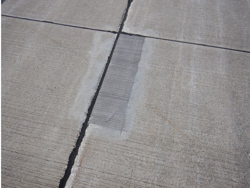
R12SP-01. Small Patching (Sample Unit No. 03).
