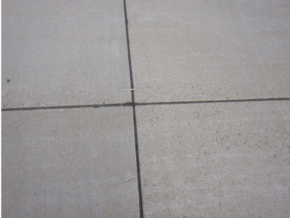
A01SX-01. Joint Seal Damage (Sample Unit No. 47).
