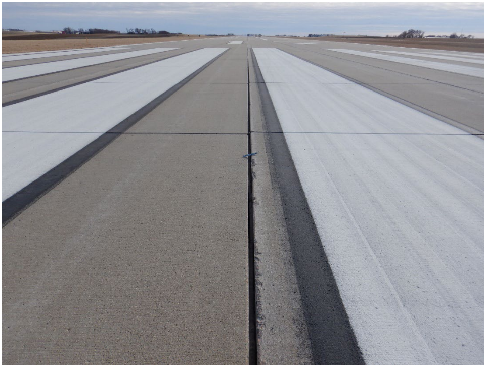
R17SX-02. Faulting (Additional Sample Unit No. 03).
