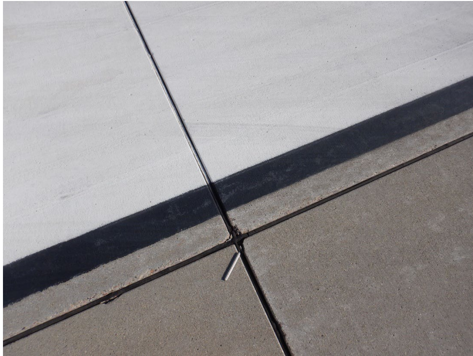
R17SX-01. Joint Seal Damage (Sample Unit No. 78).
