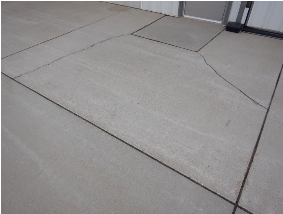
A01SX-01. LTD Cracking (Additional Sample Unit No. 56).
