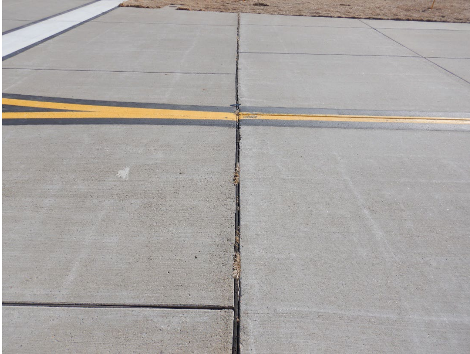
TDSX-01. Faulting (Sample Unit No. 01).
