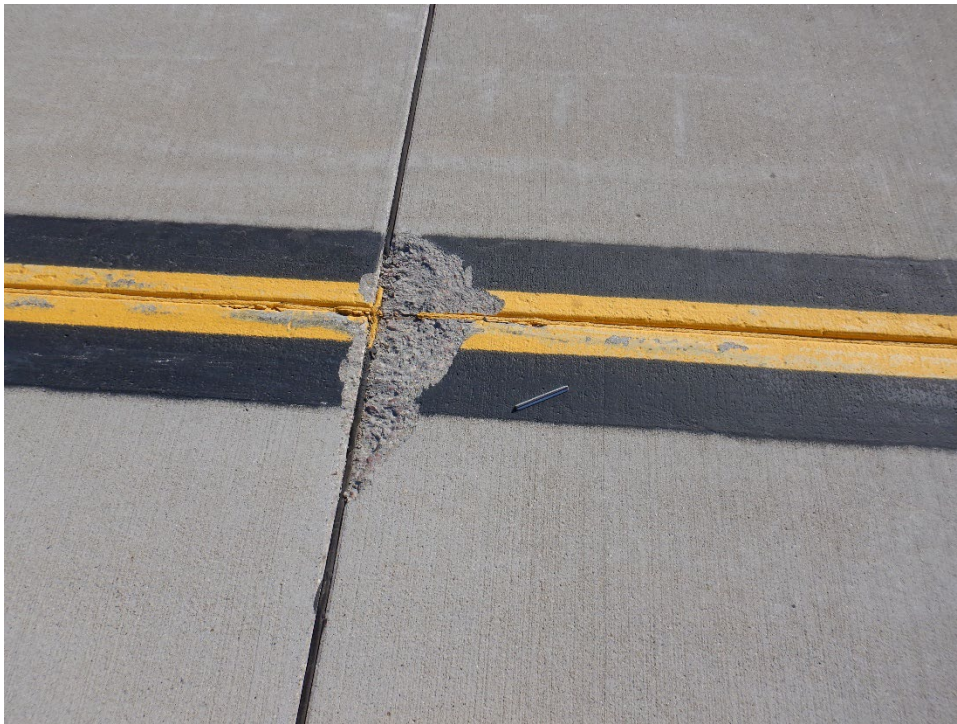
TDSX-01. Corner Spalling (Sample Unit No. 02).
