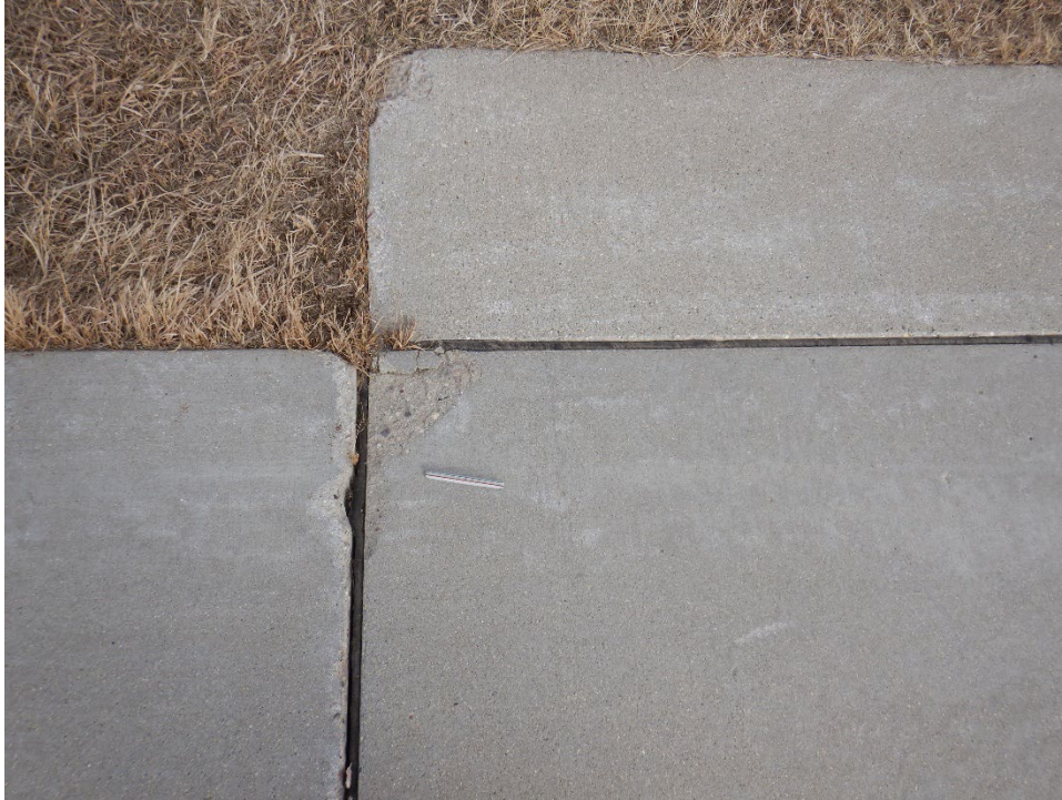
TASX-01. Corner Spalling (Sample Unit No. 06).
