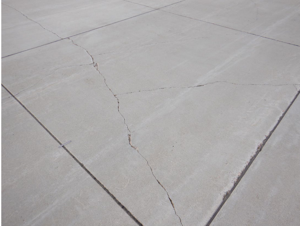
A01SX-01. Shattered Slab (Additional Sample Unit No. 41).
