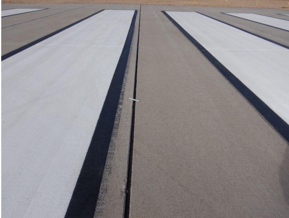
R17SX-02. Faulting (Additional Sample Unit No. 01).
