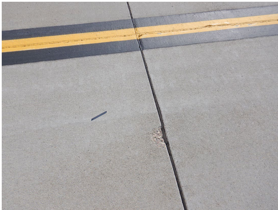
TCSX-01. Joint Spalling (Sample Unit No. 02).
