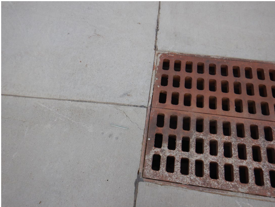
A01SX-02. Corner Spalling (Sample Unit No. 12).
