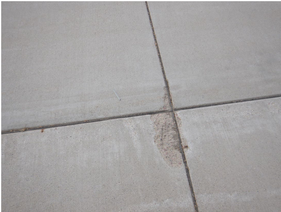
TH01SX-01. Joint Spalling (Sample Unit No. 26).
