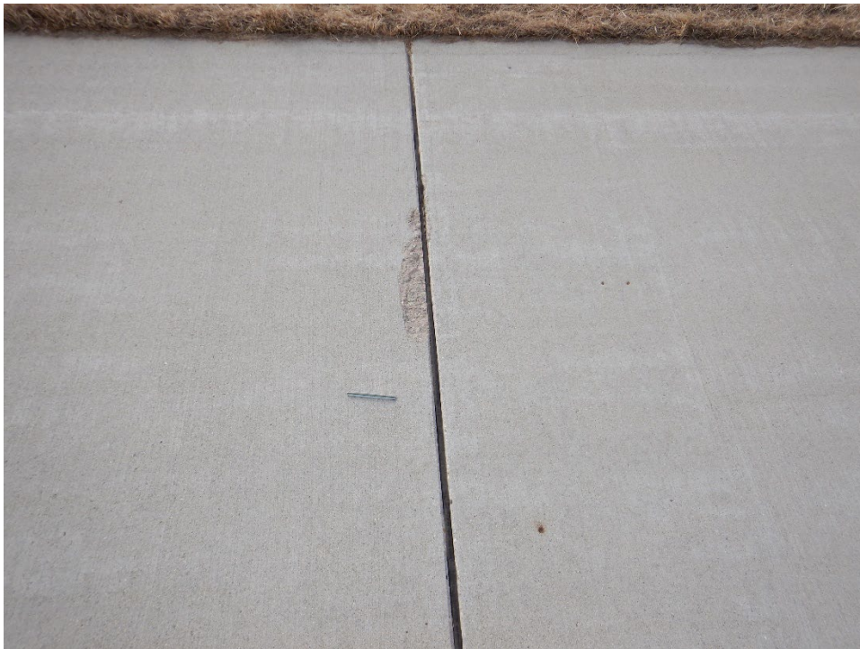
TASX-02. Joint Spalling (Sample Unit No. 02).
