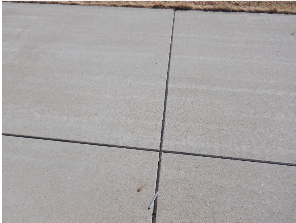
TCSX-01. Joint Seal Damage (Sample Unit No. 02).
