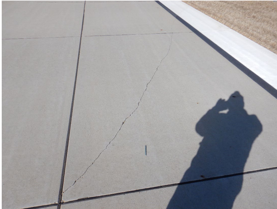
R17SX-02. LTD Cracking (Sample Unit No. 63).
