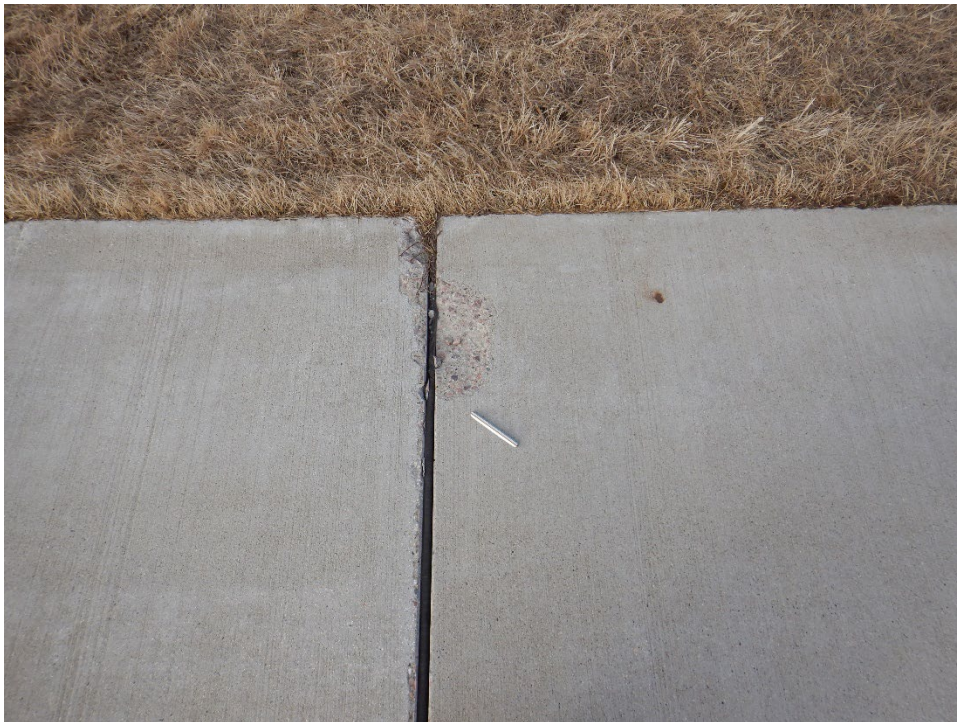
TESX-01. Joint Spalling (Sample Unit No. 06).
