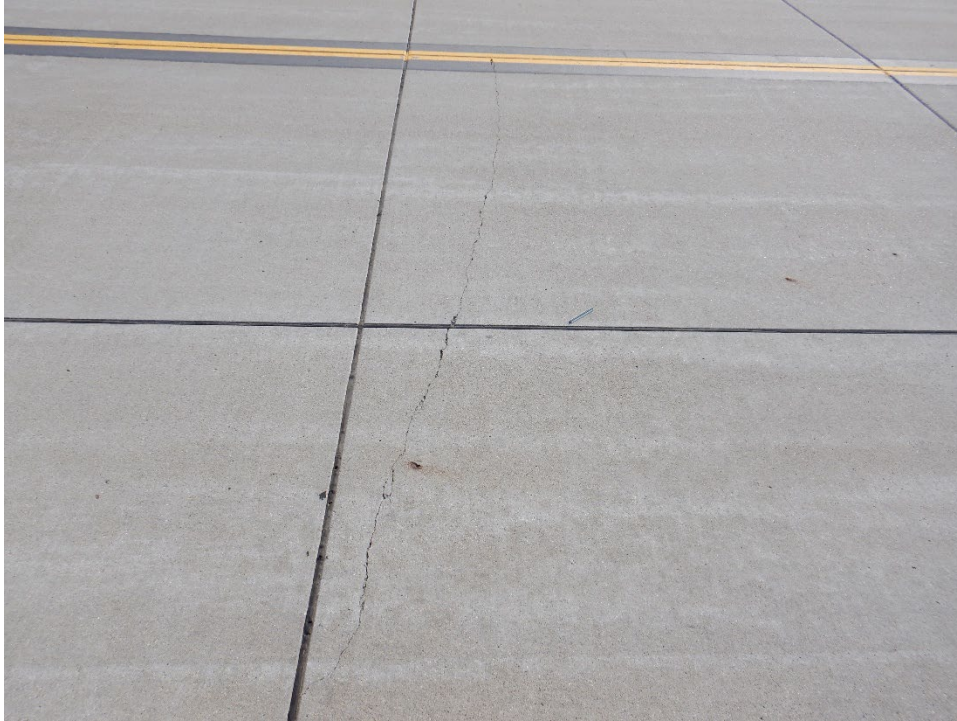
TBSX-01. LTD Cracking (Sample Unit No. 02).
