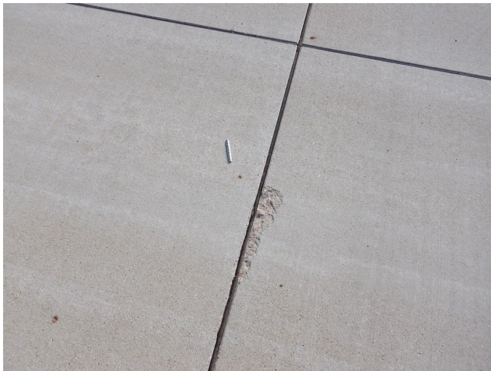
TBSX-01. Joint Spalling (Sample Unit No. 02).
