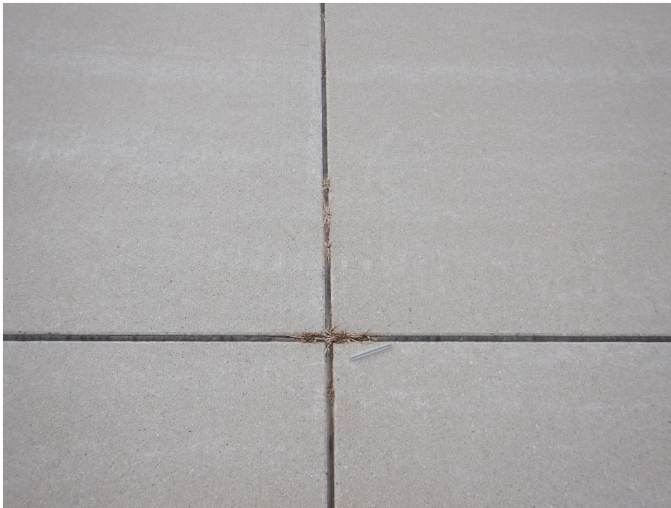
TH01SX-01. Joint Seal Damage (Sample Unit No. 11).
