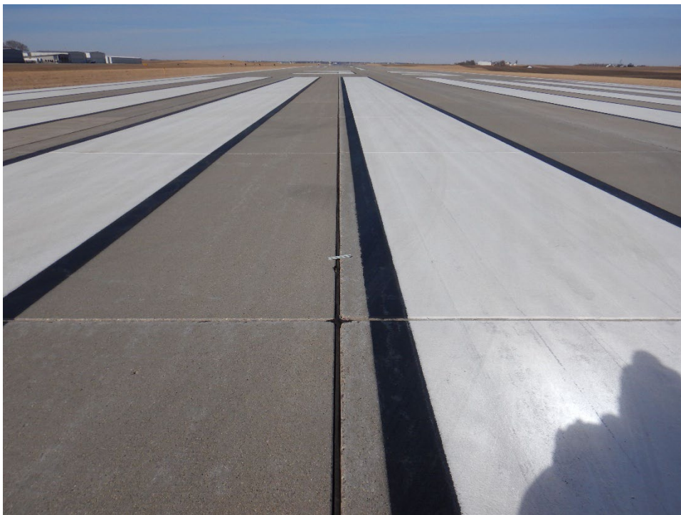
R17SX-01. Faulting (Sample Unit No. 78).
