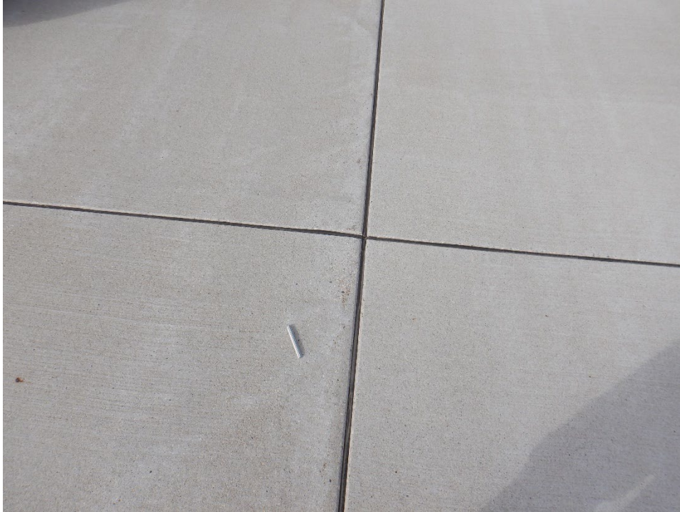
TASX-02. Joint Seal Damage (Sample Unit No. 02).
