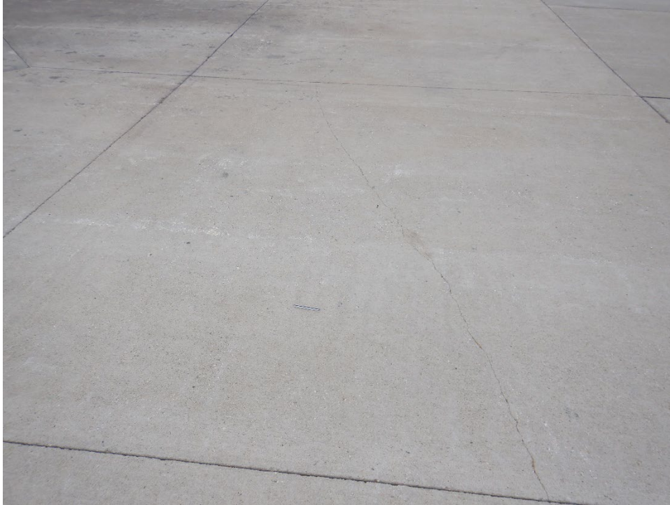
A01SX-03. LTD Cracking (Sample Unit No. 01).
