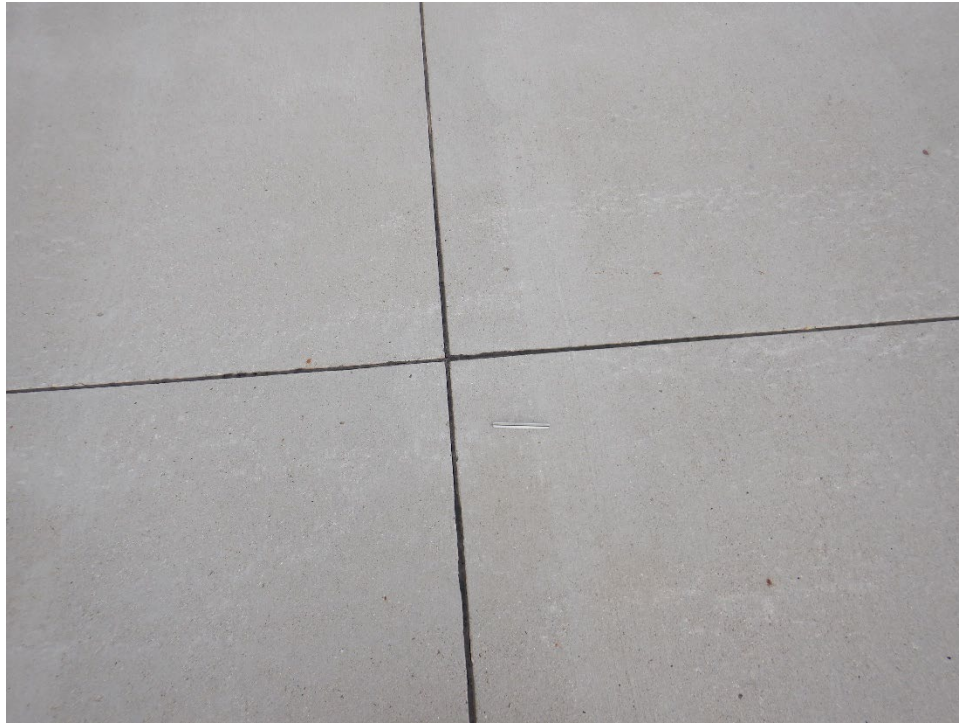
A01SX-02. Joint Seal Damage (Sample Unit No. 02).
