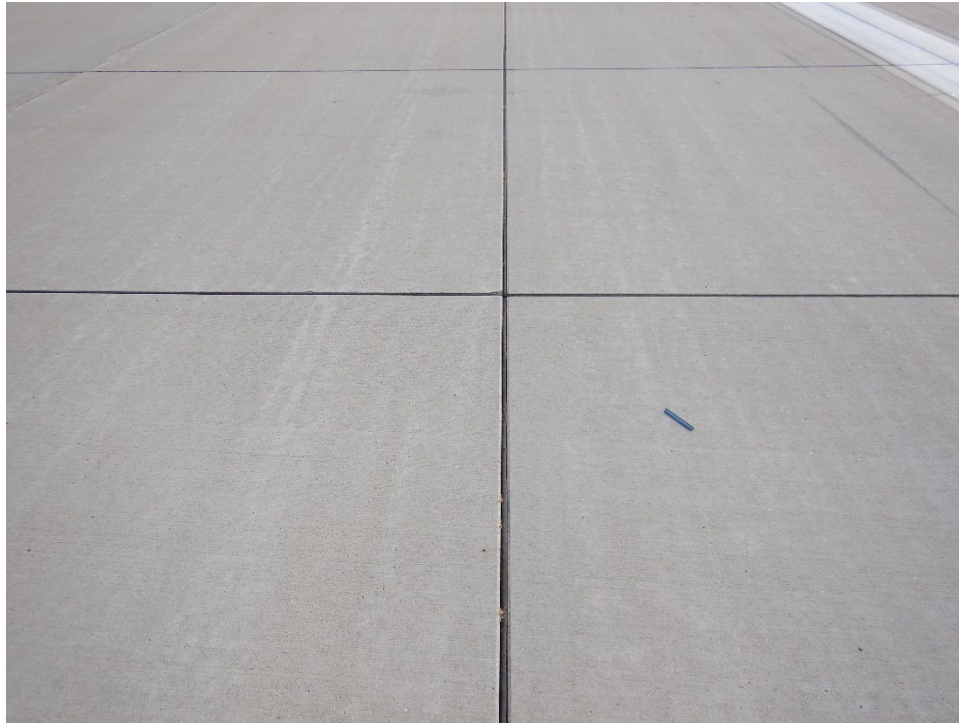
R17SX-02. Joint Seal Damage (Sample Unit No. 63).
