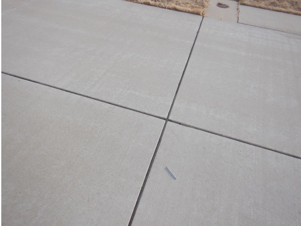
TESX-01. Joint Seal Damage (Sample Unit No. 06).
