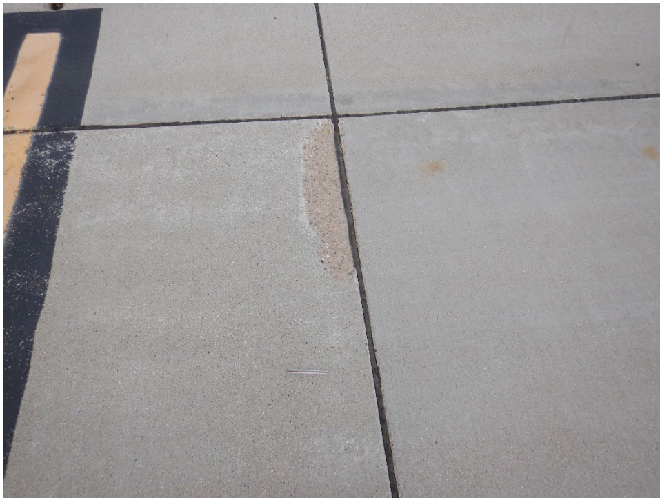
A01SX-01. Small Patching (Additional Sample Unit No. 14).
