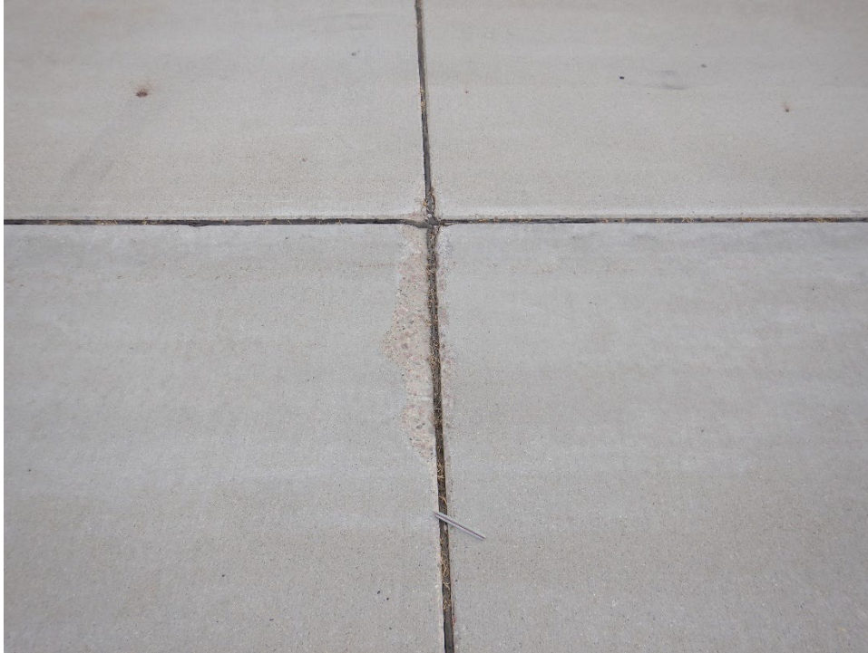
TH01SX-01. Joint Spalling (Additional Sample Unit No. 07).
