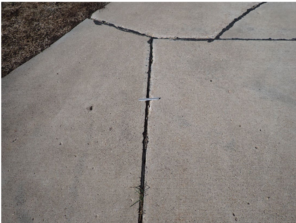
T03IS-02. Faulting (Sample Unit No. 01) (2).
