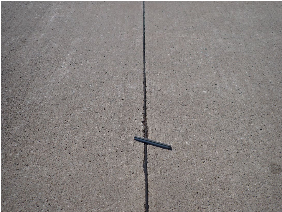
T03IS-01. Joint Seal Damage (Sample Unit No. 01).
