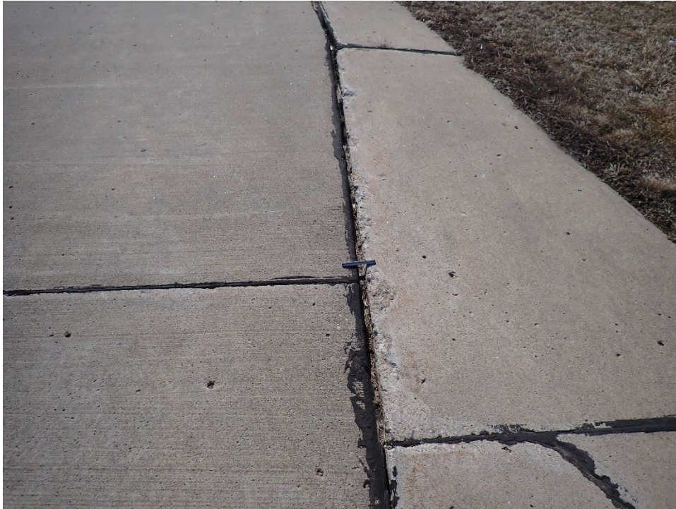
T03IS-02. Faulting (Sample Unit No. 01) (1).
