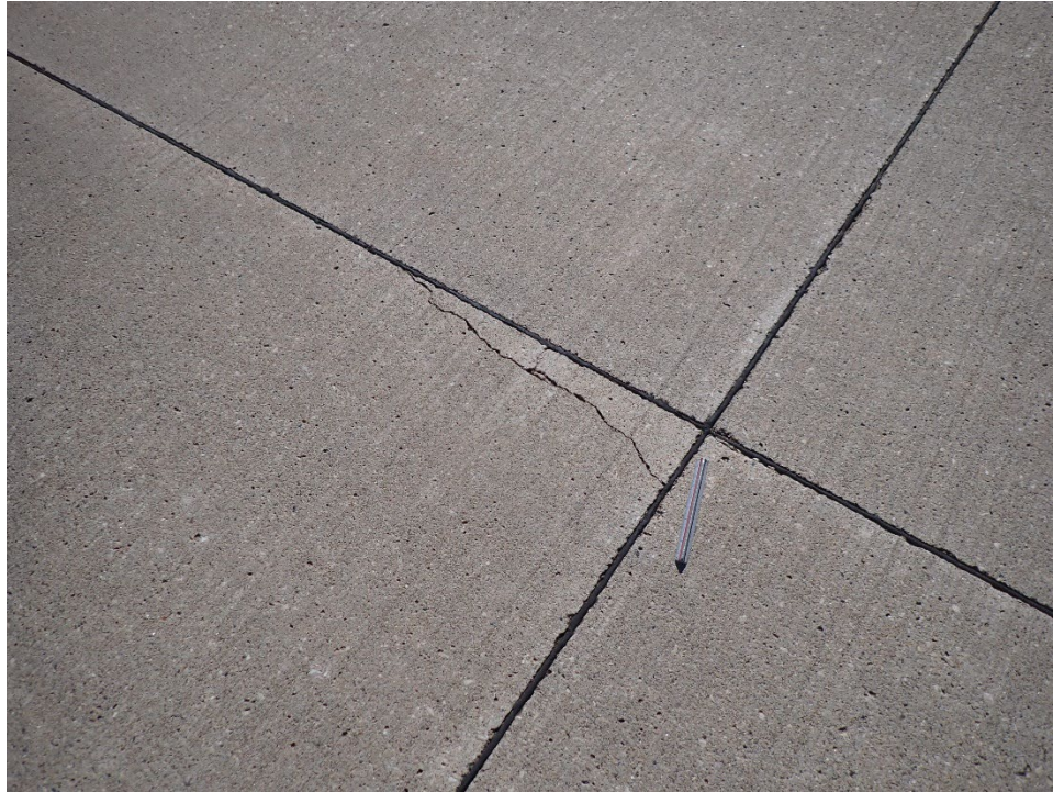
T03IS-01. Joint Spalling (Sample Unit No. 01).
