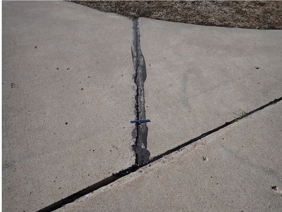
T03IS-02. LTD Cracking (Sample Unit No. 01).
