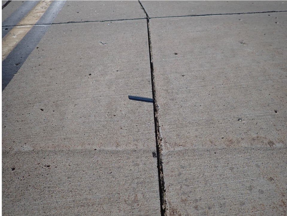
T04IS-01. Joint Seal Damage (Sample Unit No. 02).
