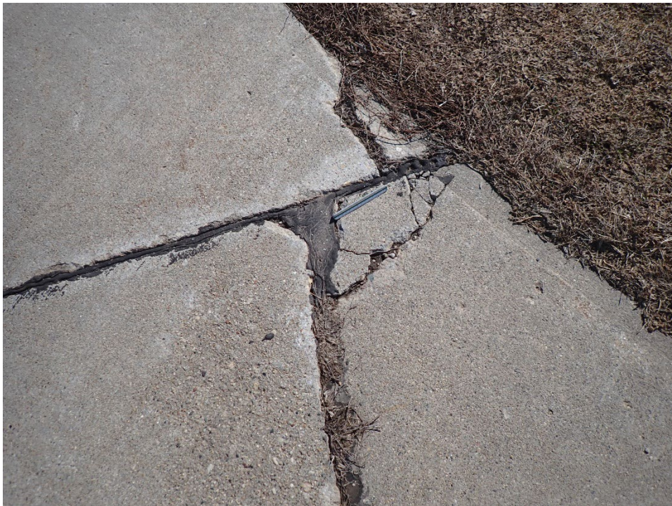
T01IS-01. Joint Spalling (Sample Unit No. 01).
