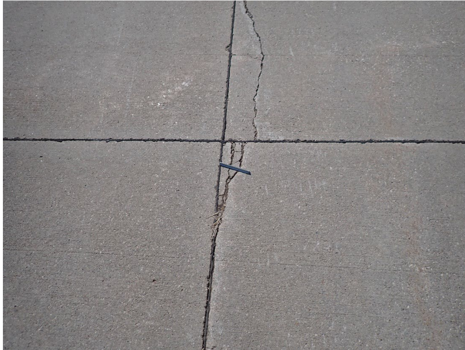
T02IS-01. Joint Spalling (Sample Unit No. 04).
