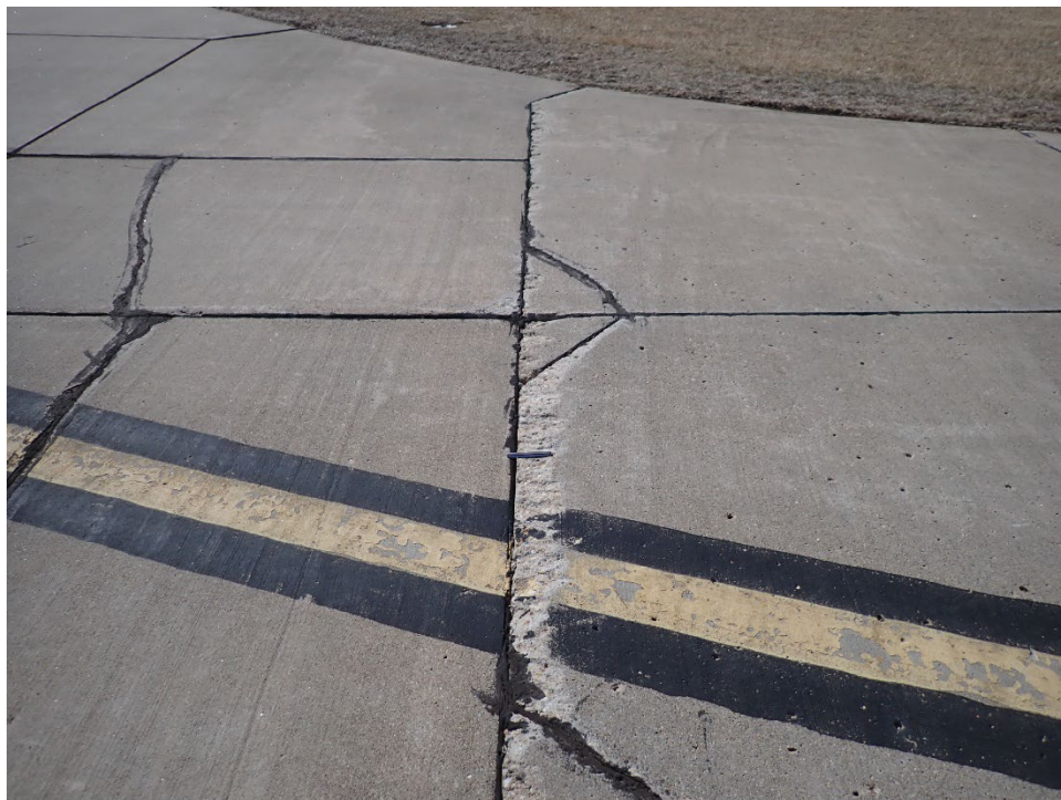
T03IS-04. Faulting (Sample Unit No. 03).
