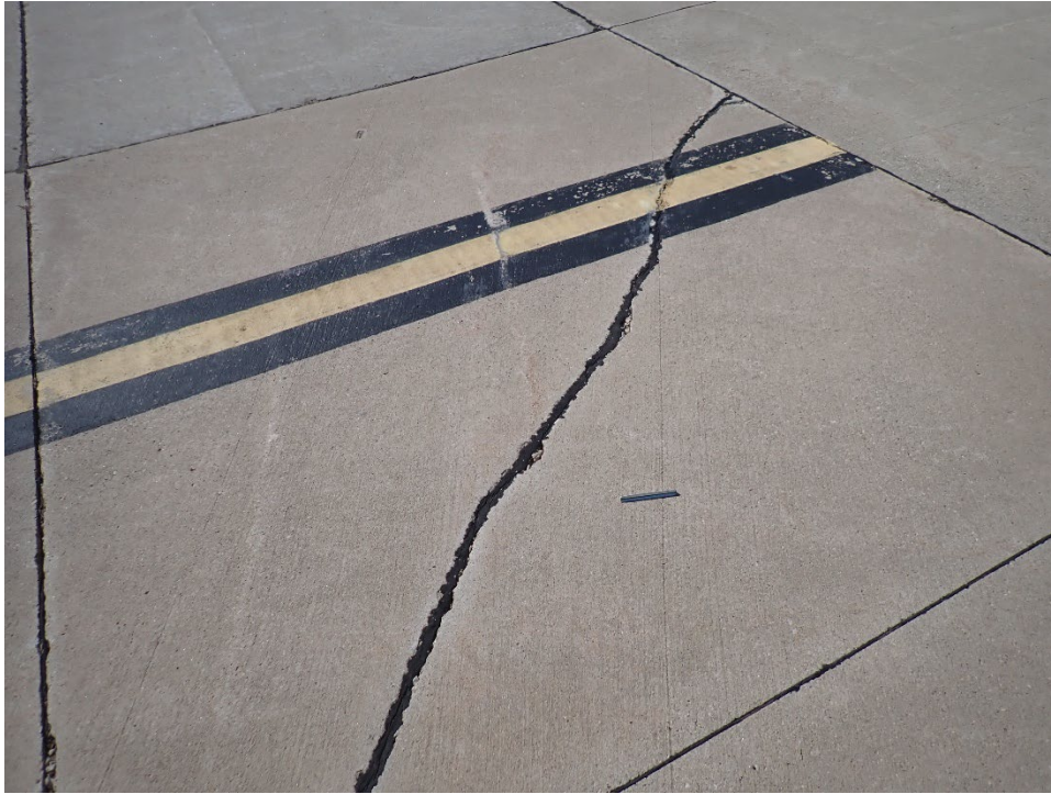
T01IS-01. LTD Cracking (Sample Unit No. 01).
