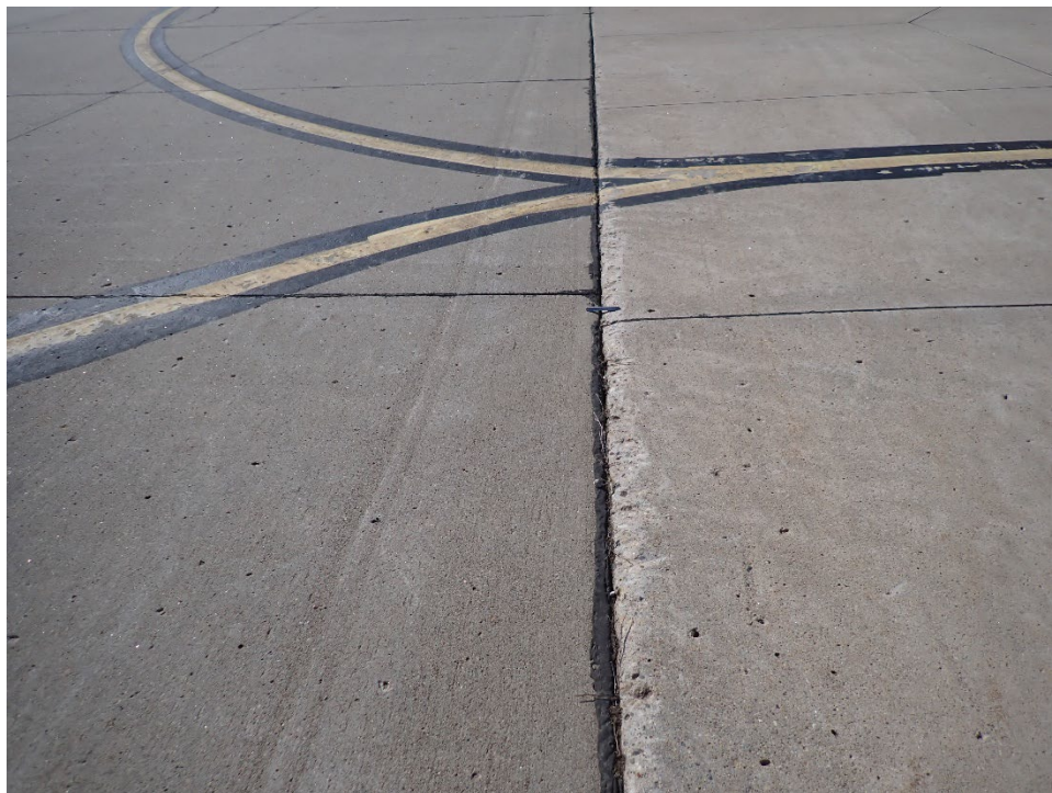
R17IS-01. Faulting (Sample Unit No. 12).
