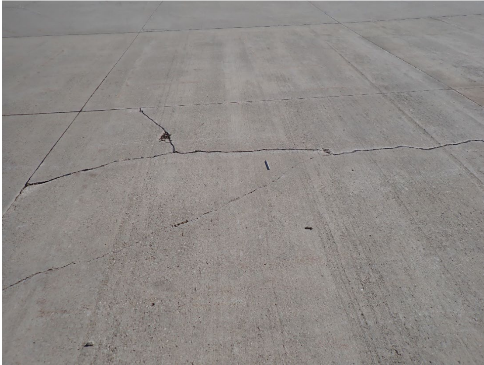
A01IS-01. Shattered Slab (Sample Unit No. 02).
