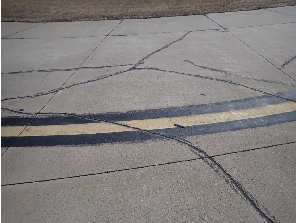
T03IS-04. Shattered Slab (Sample Unit No. 01).
