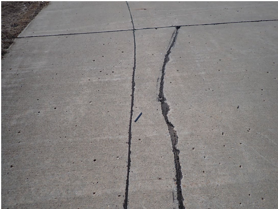
T03IS-03. LTD Cracking (Sample Unit No. 03).
