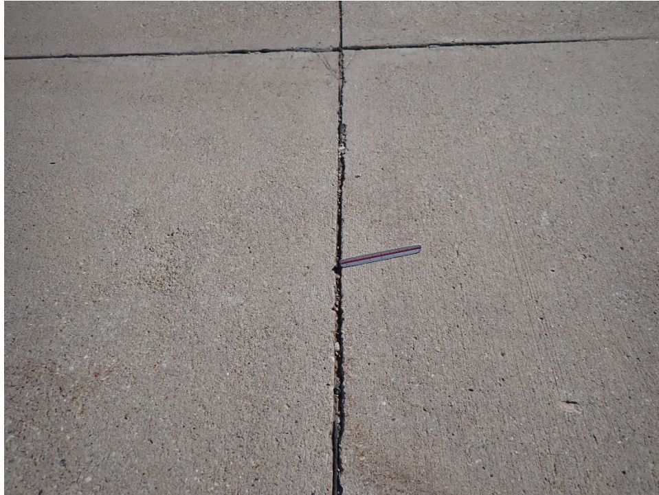
A01IS-01. Joint Seal Damage (Sample Unit No. 06).
