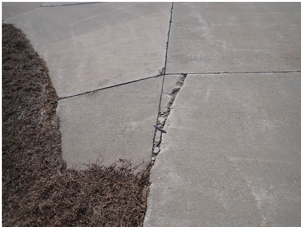
A01IS-01. Joint Spalling (Sample Unit No. 05).
