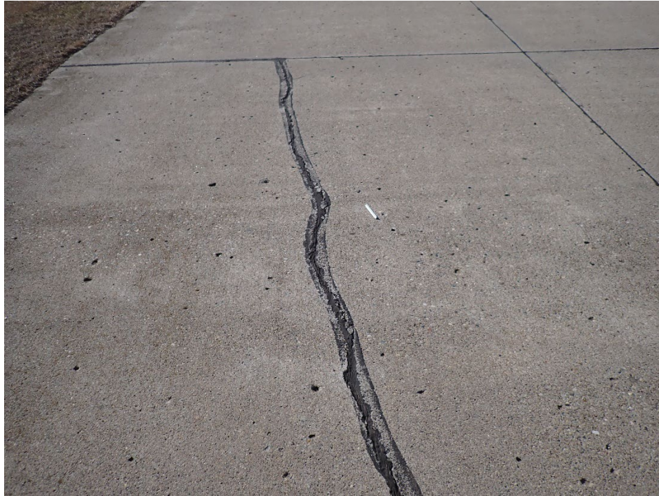
R17IS-01. LTD Cracking (Sample Unit No. 37).
