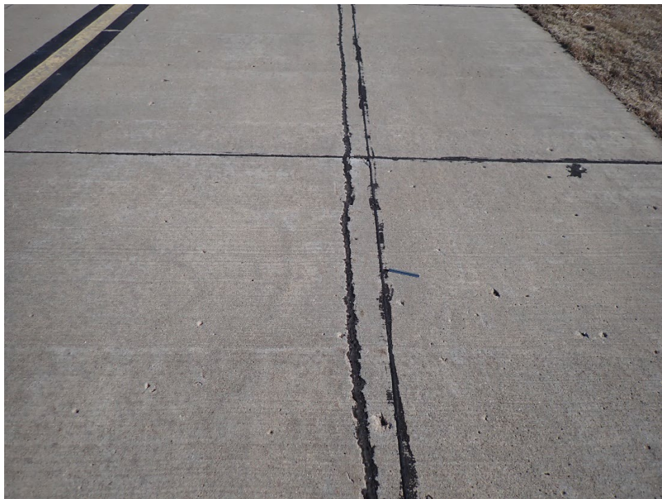
T04IS-01. LTD Cracking (Sample Unit No. 05).
