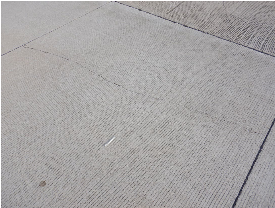
A01SD-02. LTD Cracking (Sample Unit No. 02).
