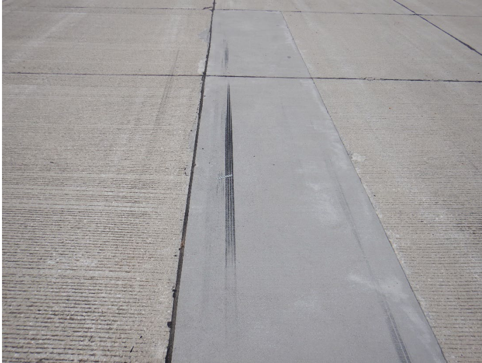
R15SD-04. Large Patching (Sample Unit No. 01).
