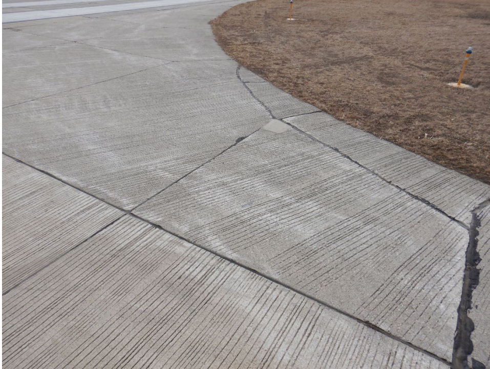
TA1SD-01. LTD Cracking (Sample Unit No. 01).
