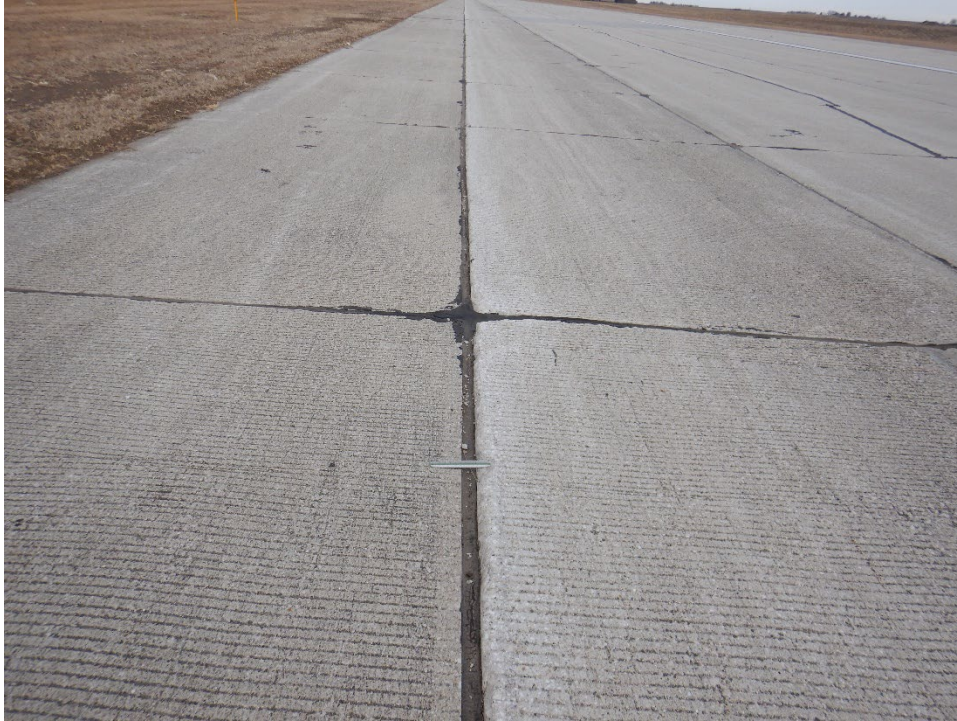
R15SD-03. Faulting (Sample Unit No. 04).
