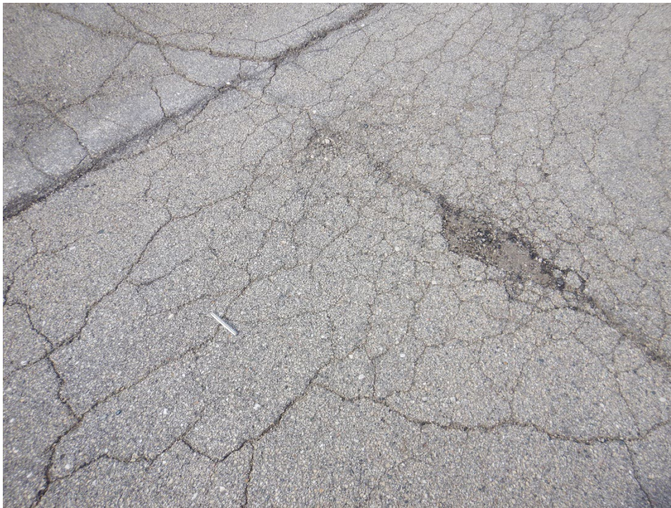
TH01SD-01. Alligator Cracking (Sample Unit No. 04).
