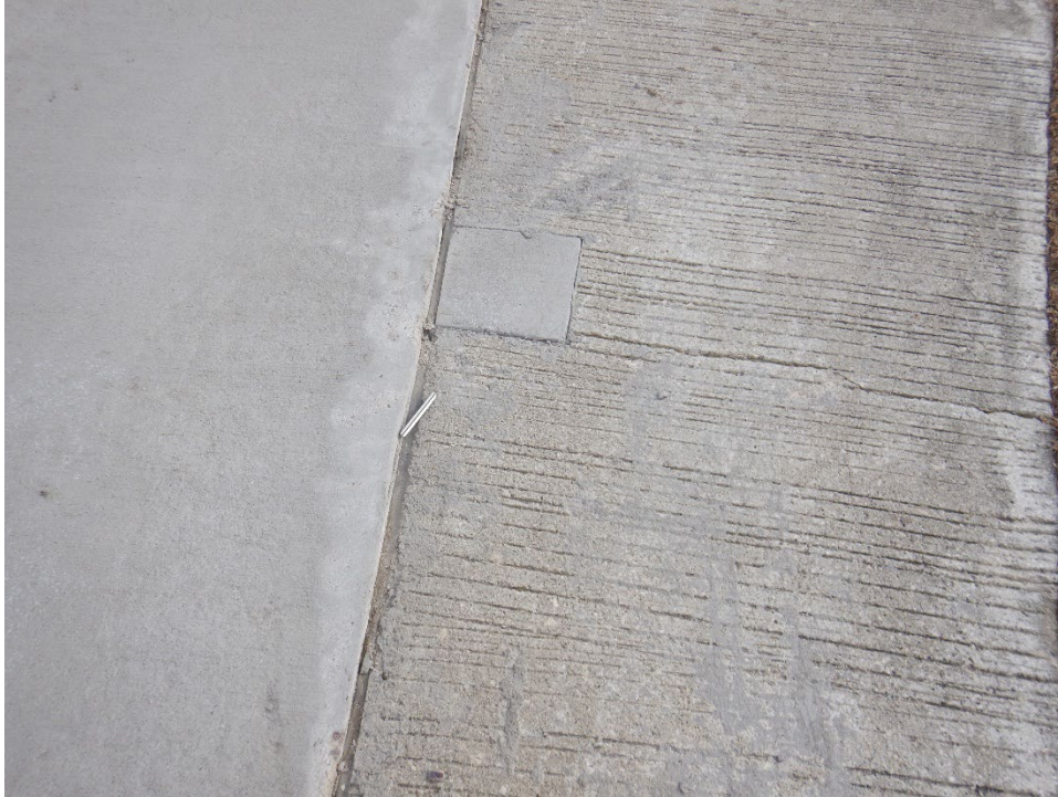
TA1SD-01. Small Patching (Sample Unit No. 02).
