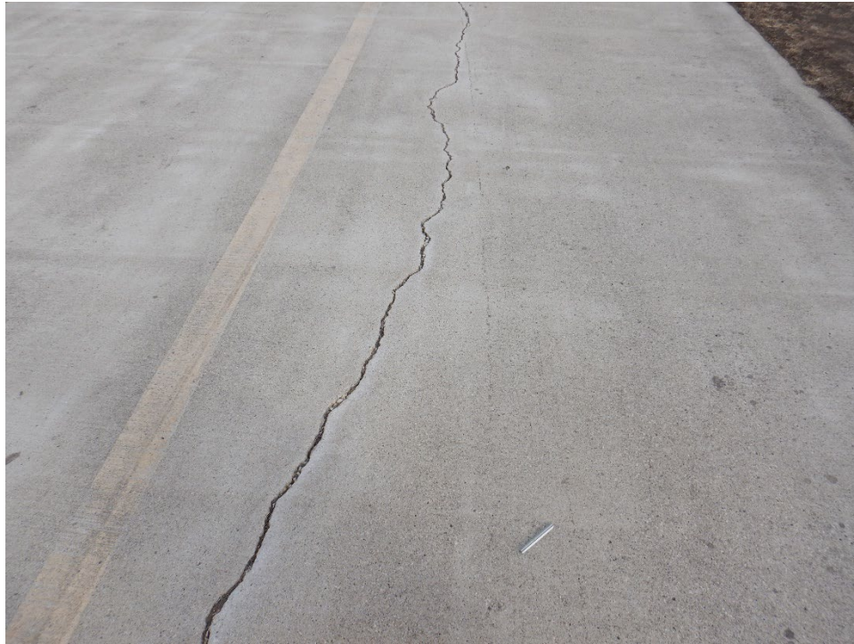
TH01SD-03. LTD Cracking (Sample Unit No. 01).
