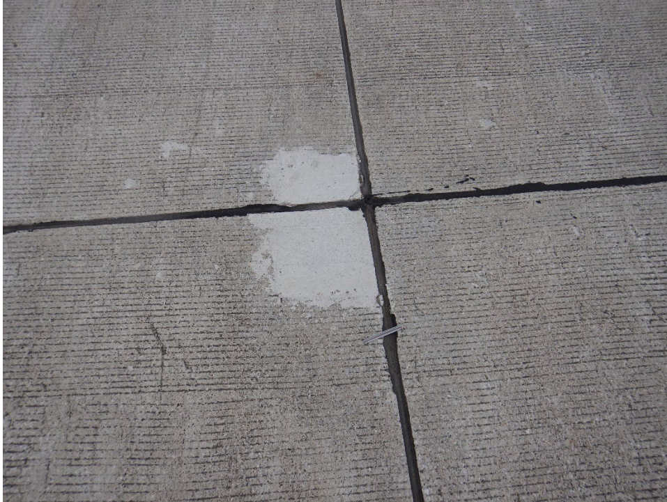
R15SD-01. Small Patching (Sample Unit No. 01).
