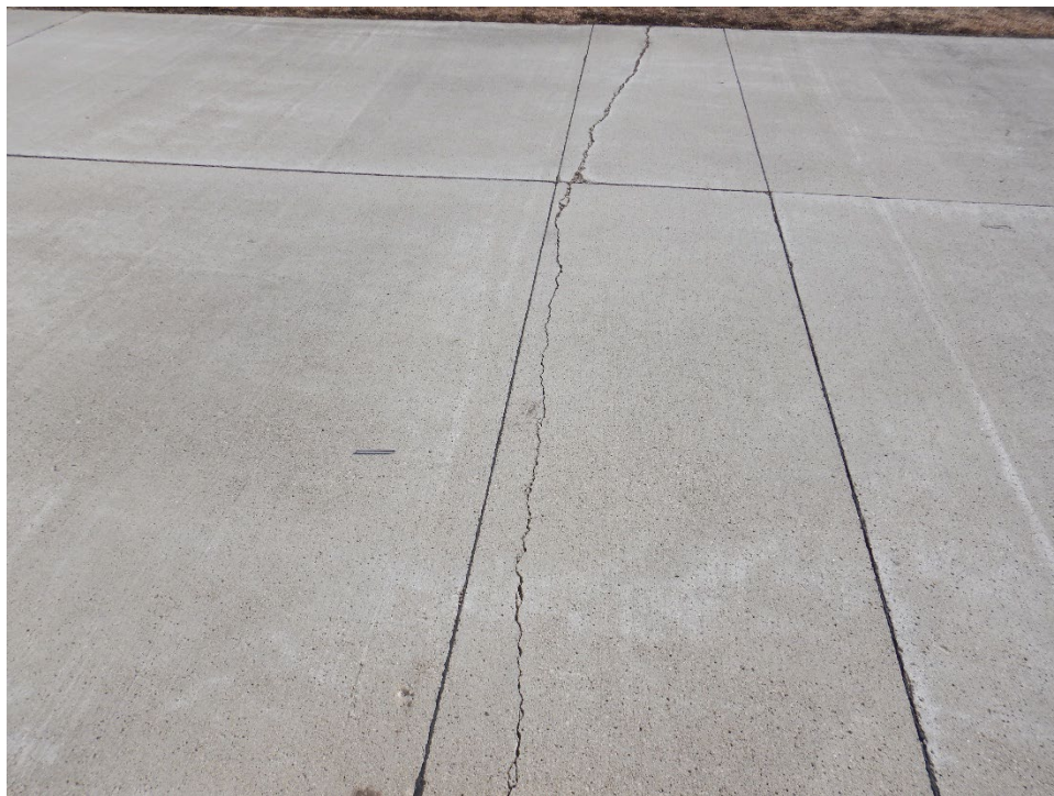
TH01SD-02. LTD Cracking (Sample Unit No. 04).
