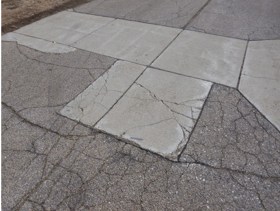
TH01SD-01. Patching (Sample Unit No. 04).
