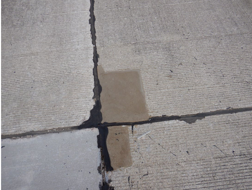
R15SD-02. Small Patching (Sample Unit No. 04).
