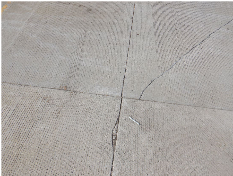
A01SD-03. Joint Seal Damage (Sample Unit No. 02).
