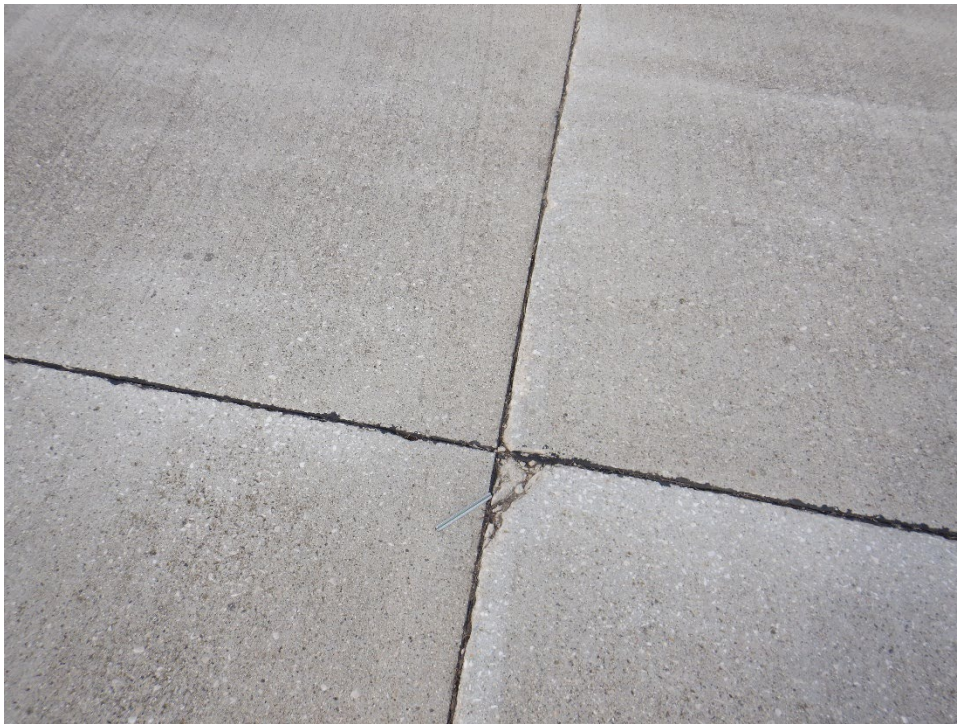
TH01SD-02. Corner Spalling (Sample Unit No. 03).
