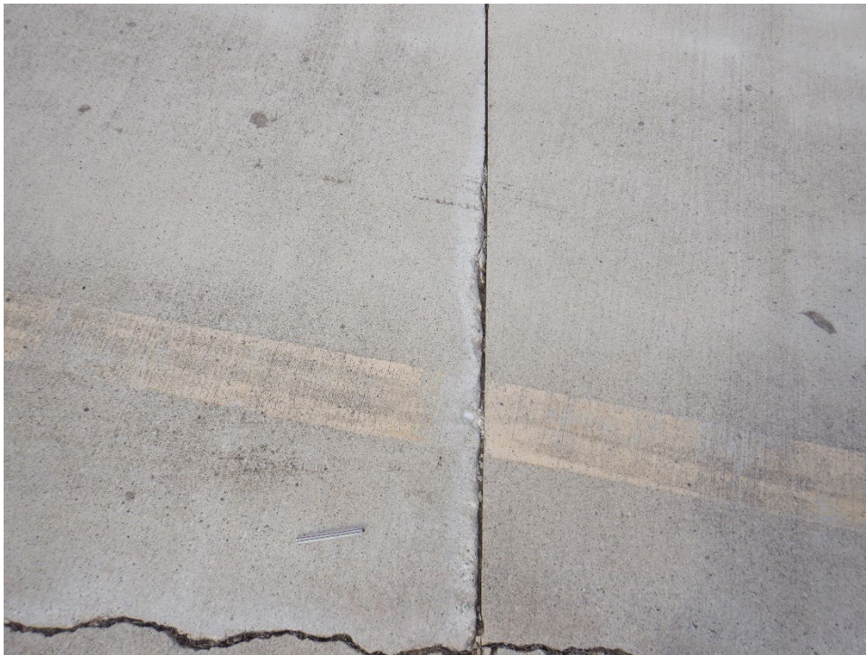
TH01SD-03. Joint Seal Damage (Sample Unit No. 01).
