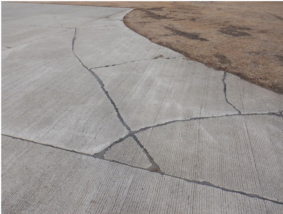
TA1SD-01. Shattered Slab (Sample Unit No. 03).
