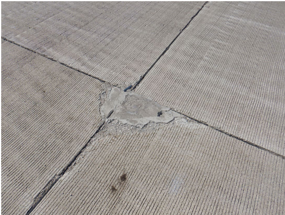
A01SD-01. Durability Cracking (Sample Unit No. 02).
