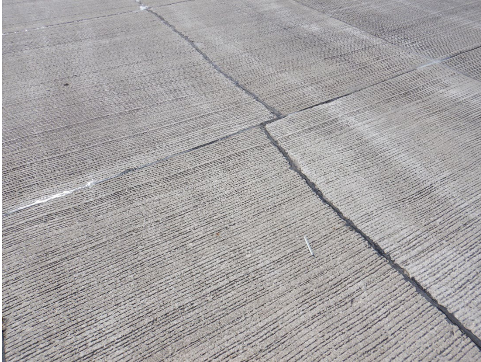
A01SD-01. LTD Cracking (Sample Unit No. 07).
