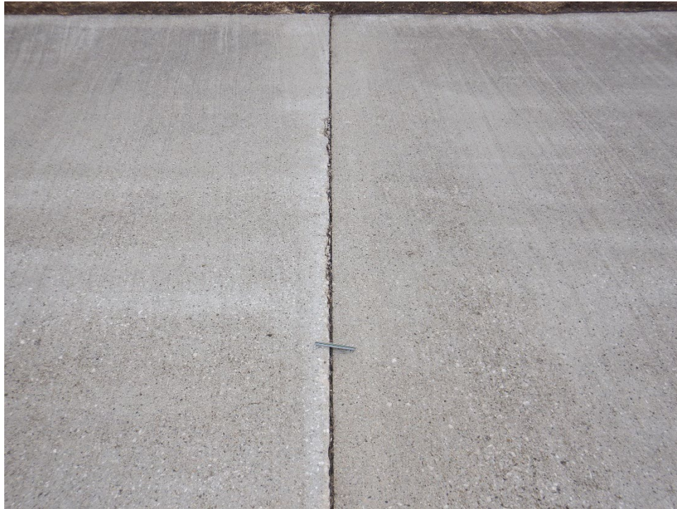
TH01SD-02. Faulting (Sample Unit No. 03).
