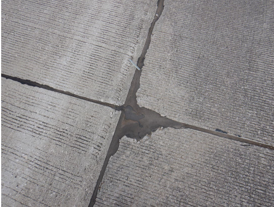
R15SD-02. Corner Spalling (Sample Unit No. 04).
