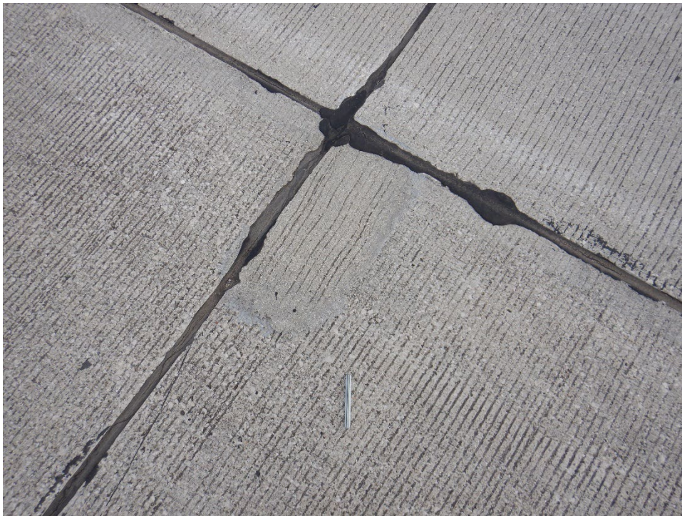
R15SD-03. Small Patching (Sample Unit No. 04).
