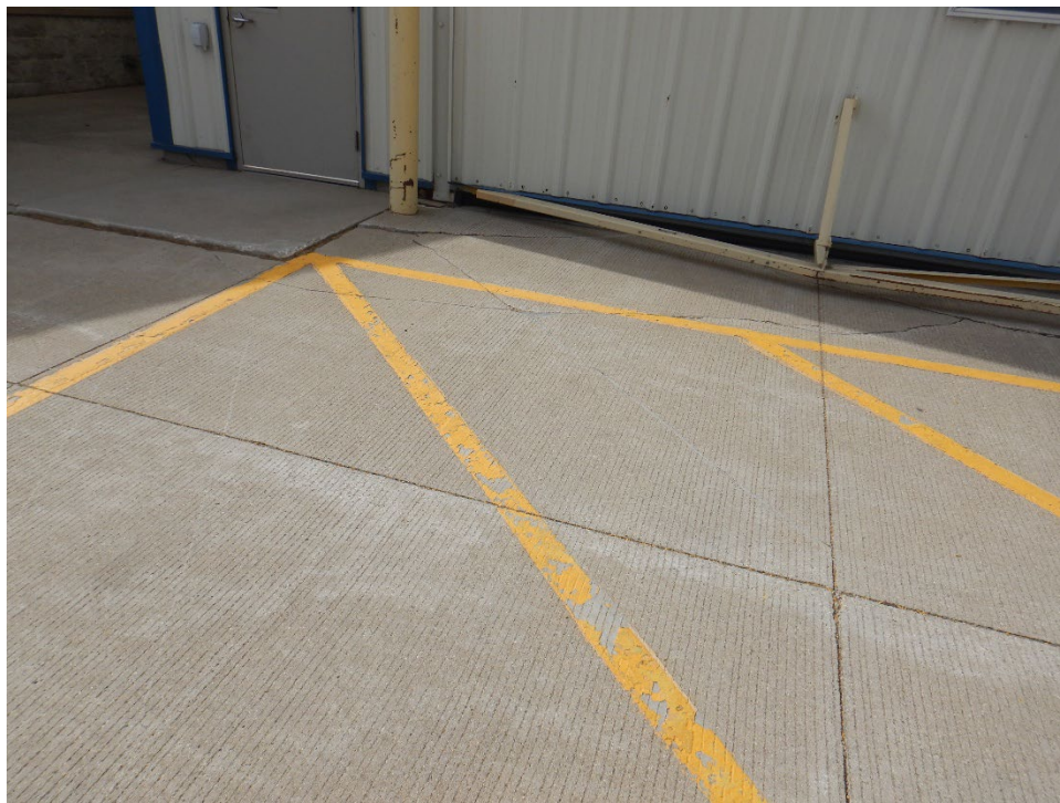
A01SD-03. Shattered Slab (Sample Unit No. 01).
