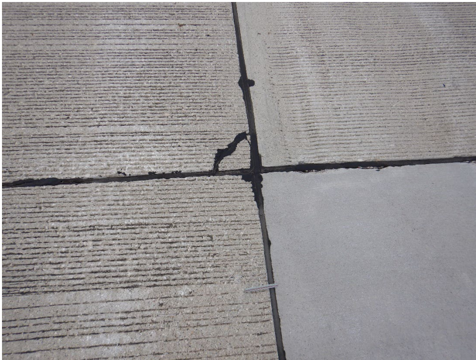
R15SD-04. Corner Spalling (Sample Unit No. 01).
