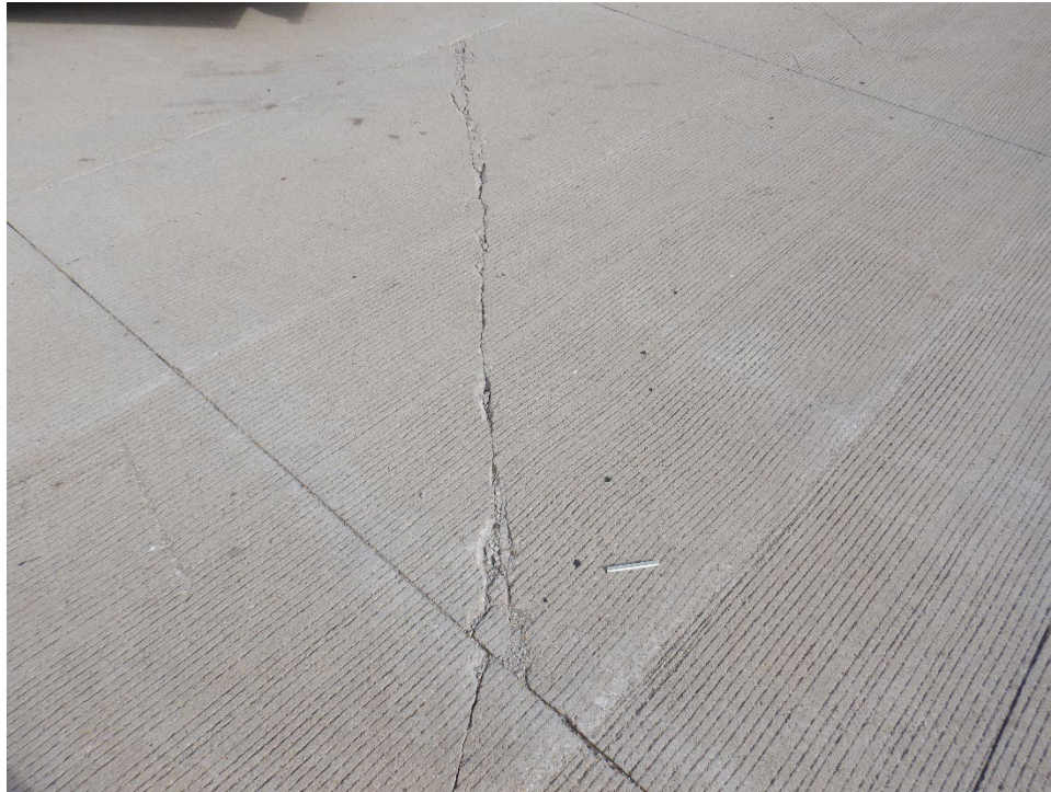
A01SD-03. LTD Cracking (Sample Unit No. 02).
