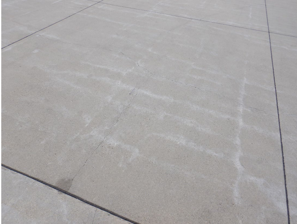
A01SD-04. Shattered Slab (Sample Unit No. 04).
