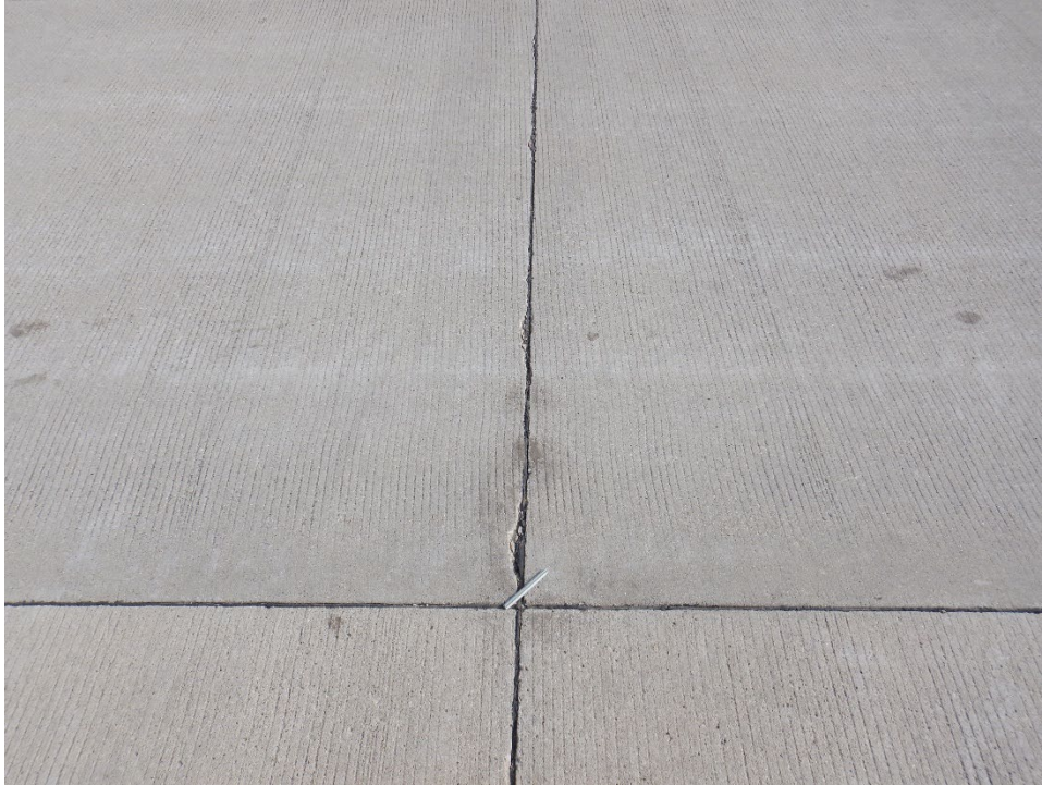
A01SD-02. Joint Seal Damage (Sample Unit No. 07).
