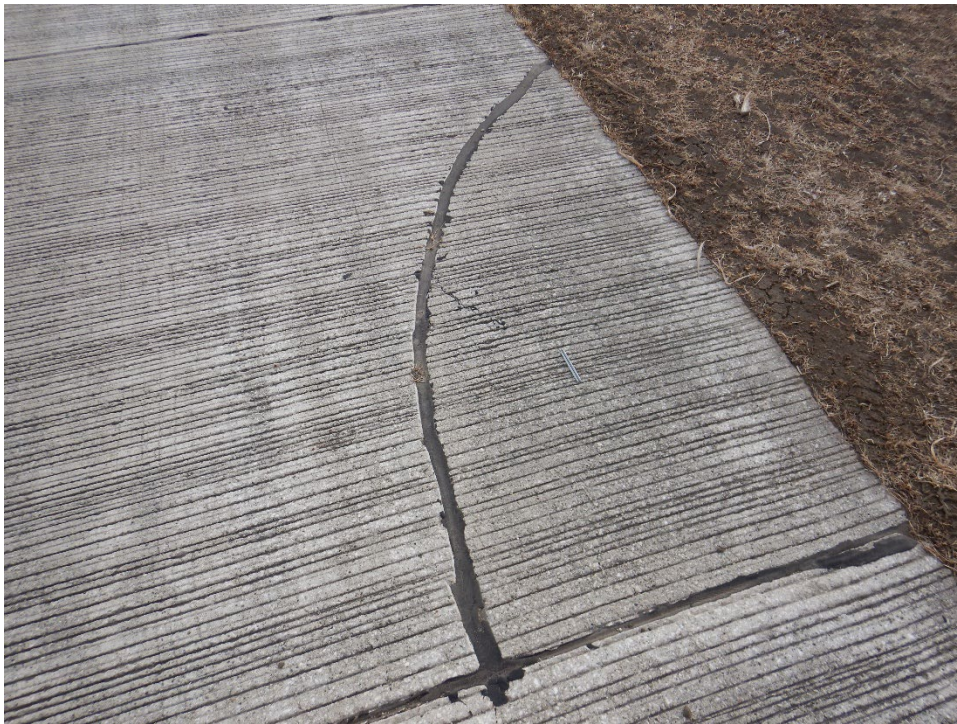
TA2SD-01. LTD Cracking (Sample Unit No. 05).
