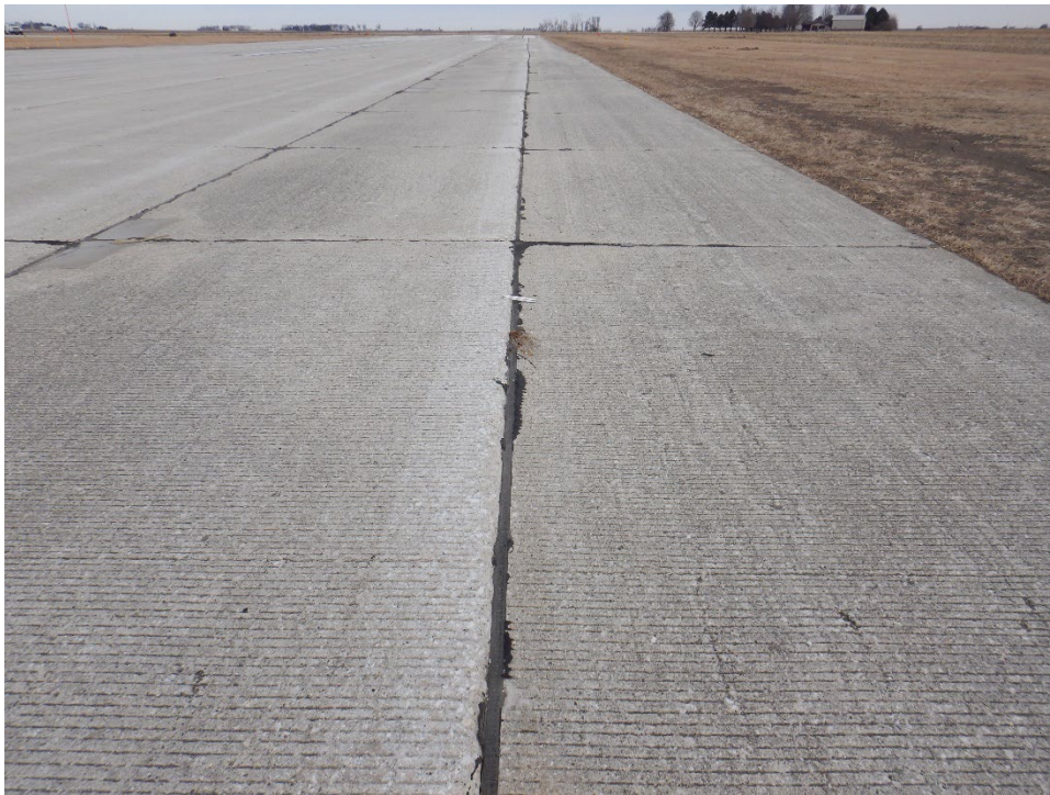
R15SD-02. Faulting (Sample Unit No. 20).
