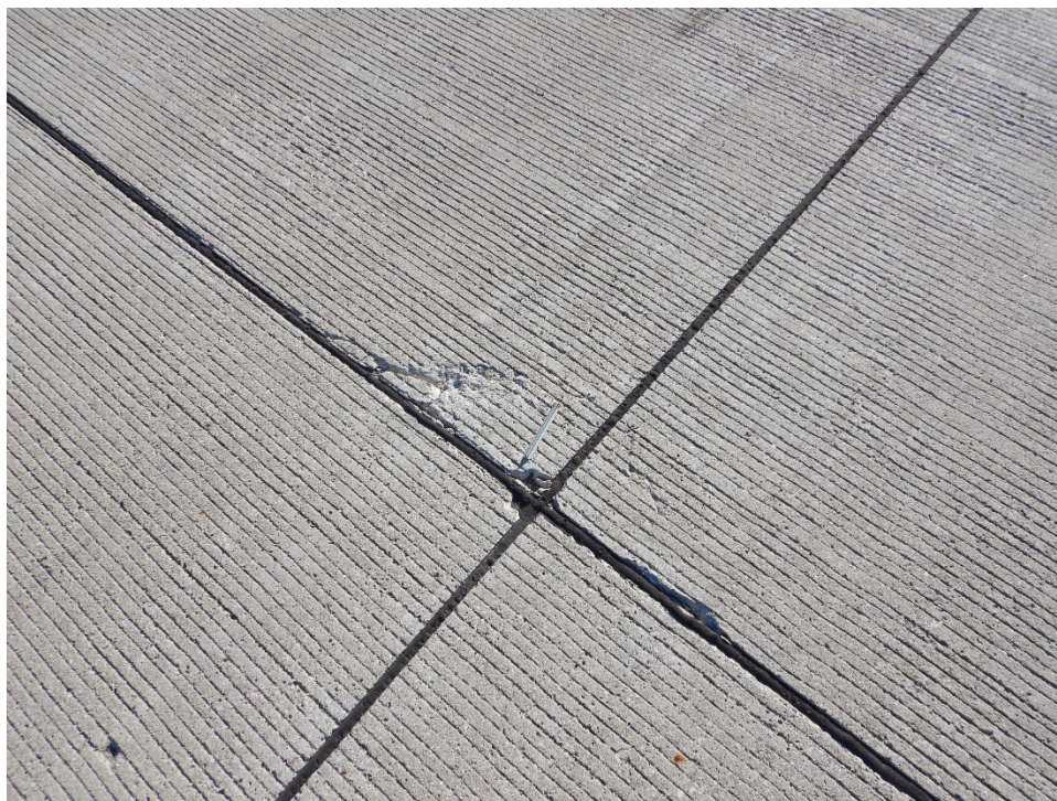
R15SD-04. Corner Spalling (Sample Unit No. 36).
