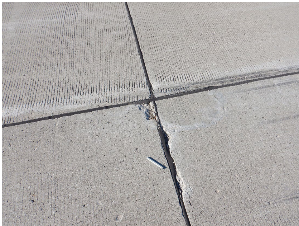
R15SD-01. Corner Spalling (Sample Unit No. 16).
