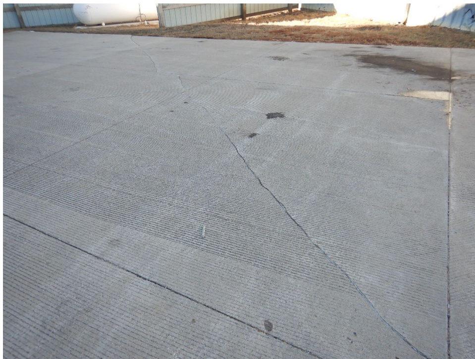
A01SD-03. LTD Cracking (Sample Unit No. 02).
