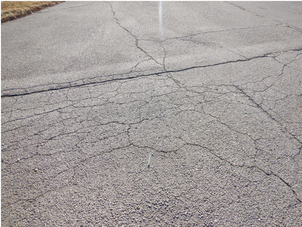
TH01SD-01. Alligator Cracking (Sample Unit No. 04).
