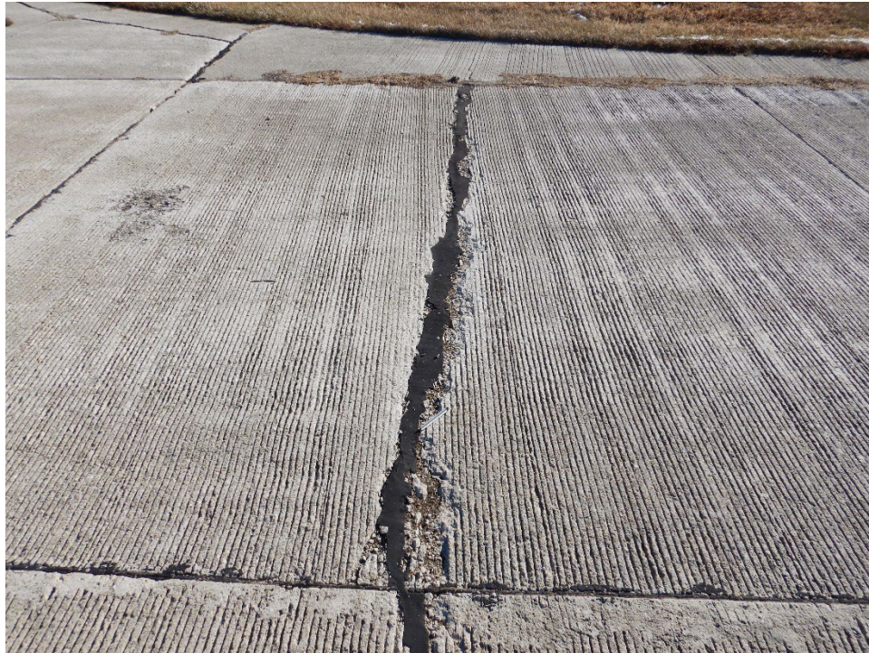
T02SD-01. LTD Cracking (Sample Unit No. 02).
