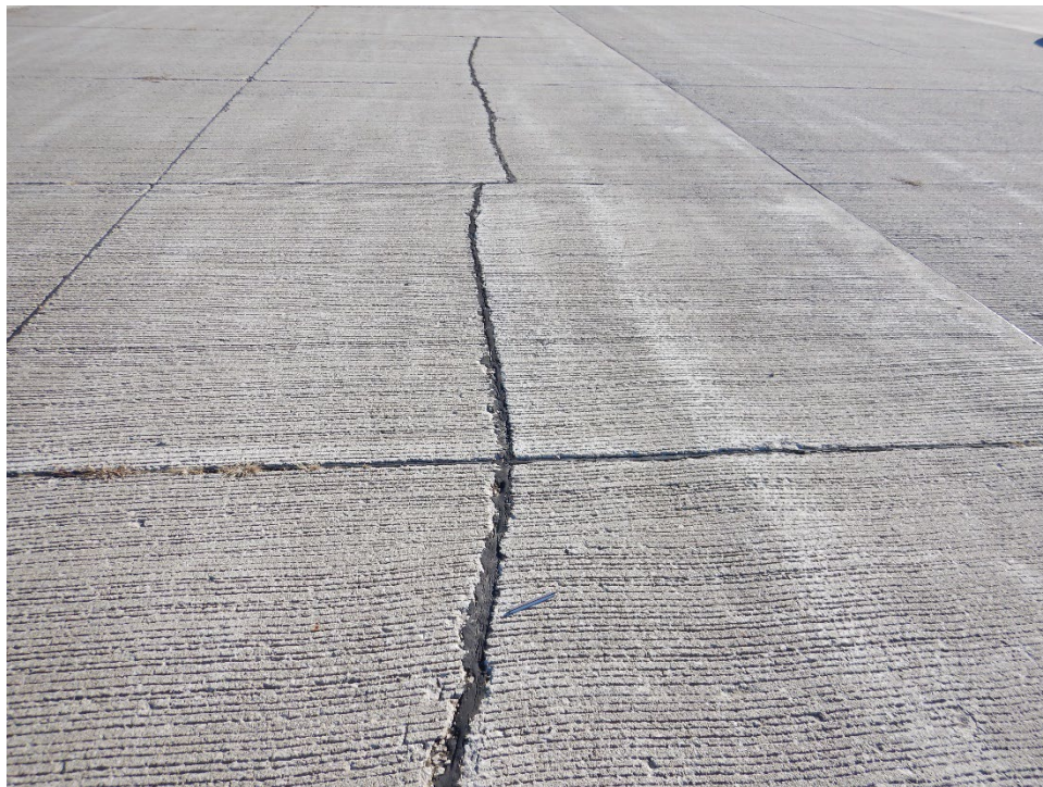
A01SD-01. LTD Cracking (Sample Unit No. 07).
