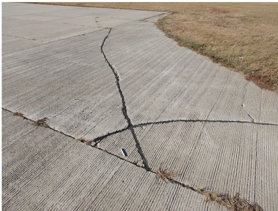
T02SD-01. Shattered Slab (Sample Unit No. 03).
