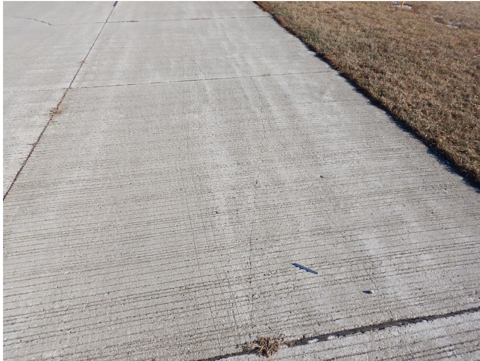
T01SD-01. LTD Cracking (Sample Unit No. 05).
