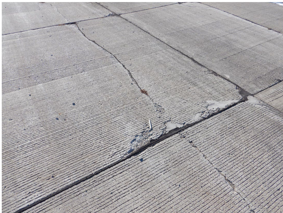
R15SD-04. Durability Cracking (Additional Sample Unit No. 06) (2).
