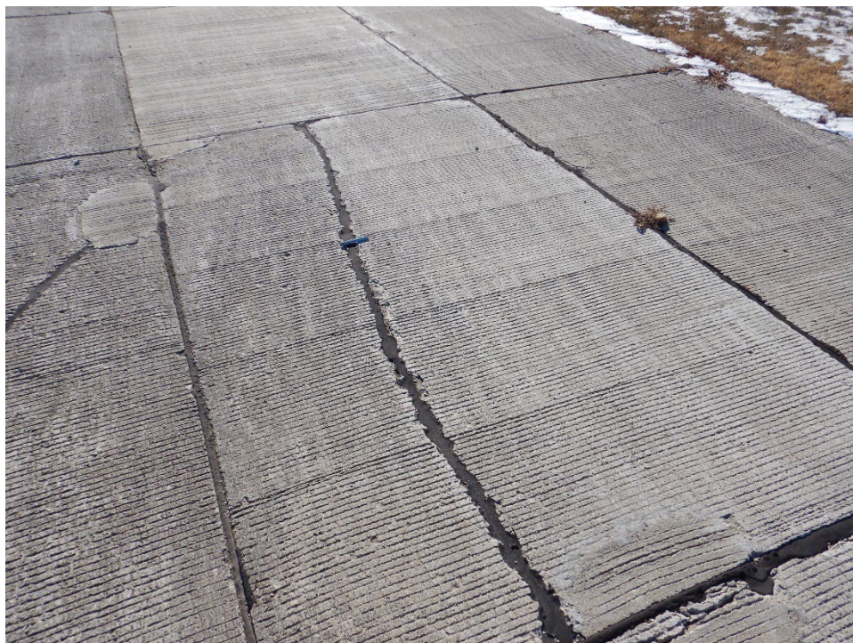
R15SD-03. LTD Cracking (Sample Unit No. 04).
