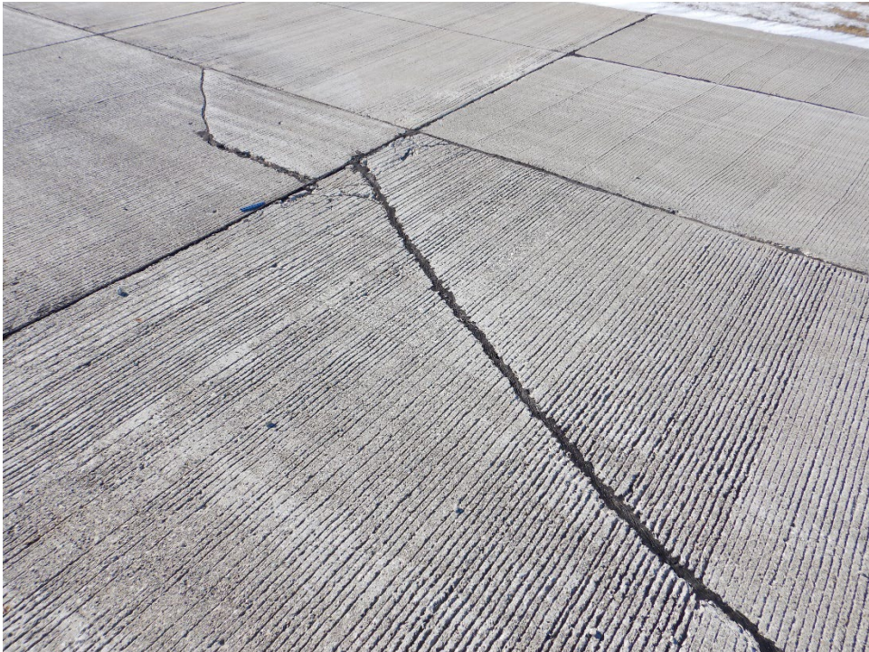
R15SD-04. LTD Cracking (Sample Unit No. 21).
