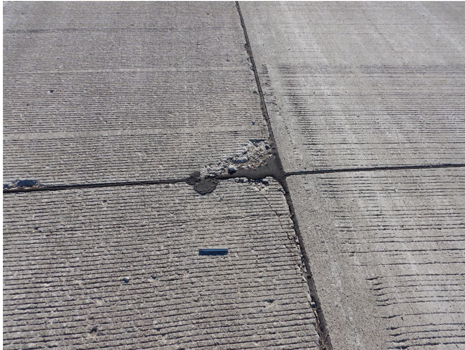
R15SD-02. Corner Spalling (Sample Unit No. 04).
