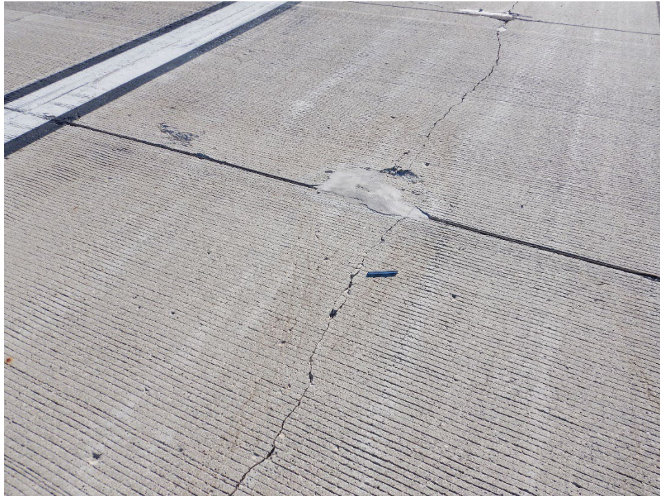
R15SD-04. Durability Cracking (Additional Sample Unit No. 06) (1).
