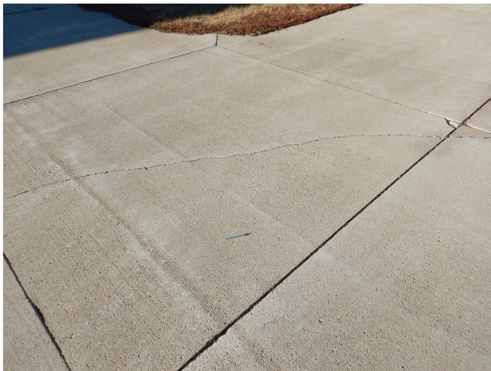
TH01SD-02. LTD Cracking (Sample Unit No. 03).
