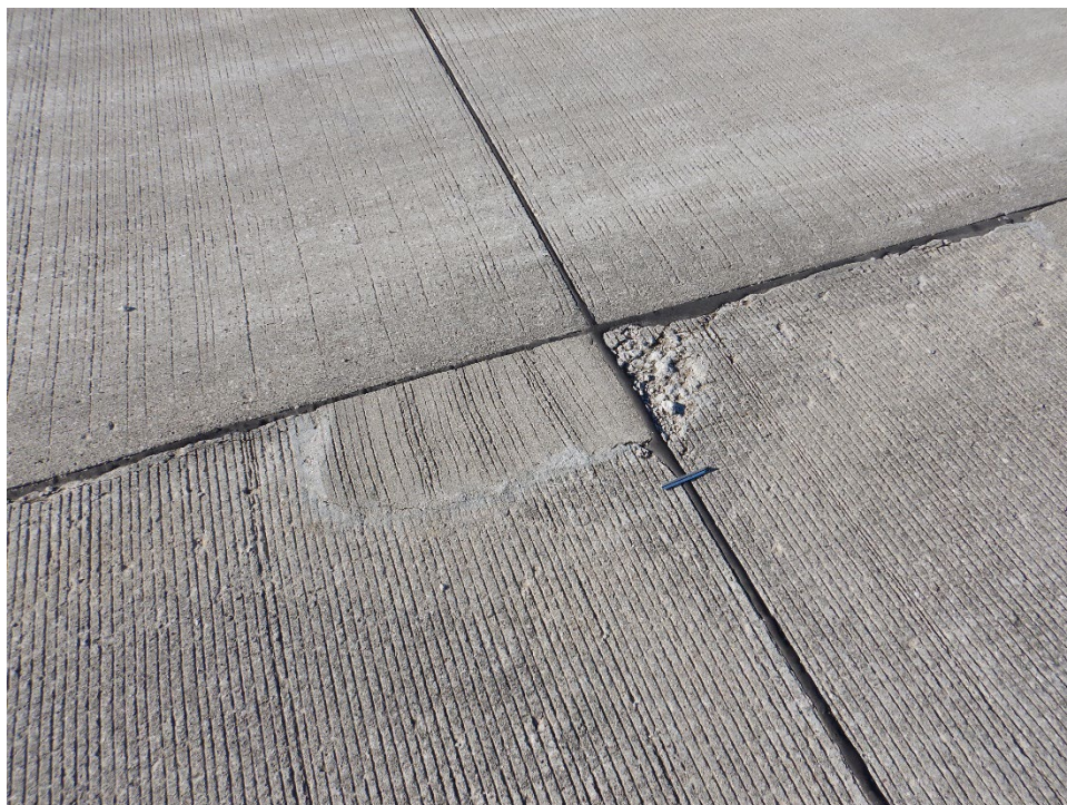
R15SD-02. Small Patching (Sample Unit No. 04).
