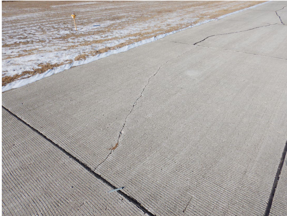
R15SD-01. LTD Cracking (Sample Unit No. 10).
