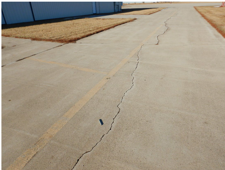
TH01SD-03. LTD Cracking (Sample Unit No. 01).
