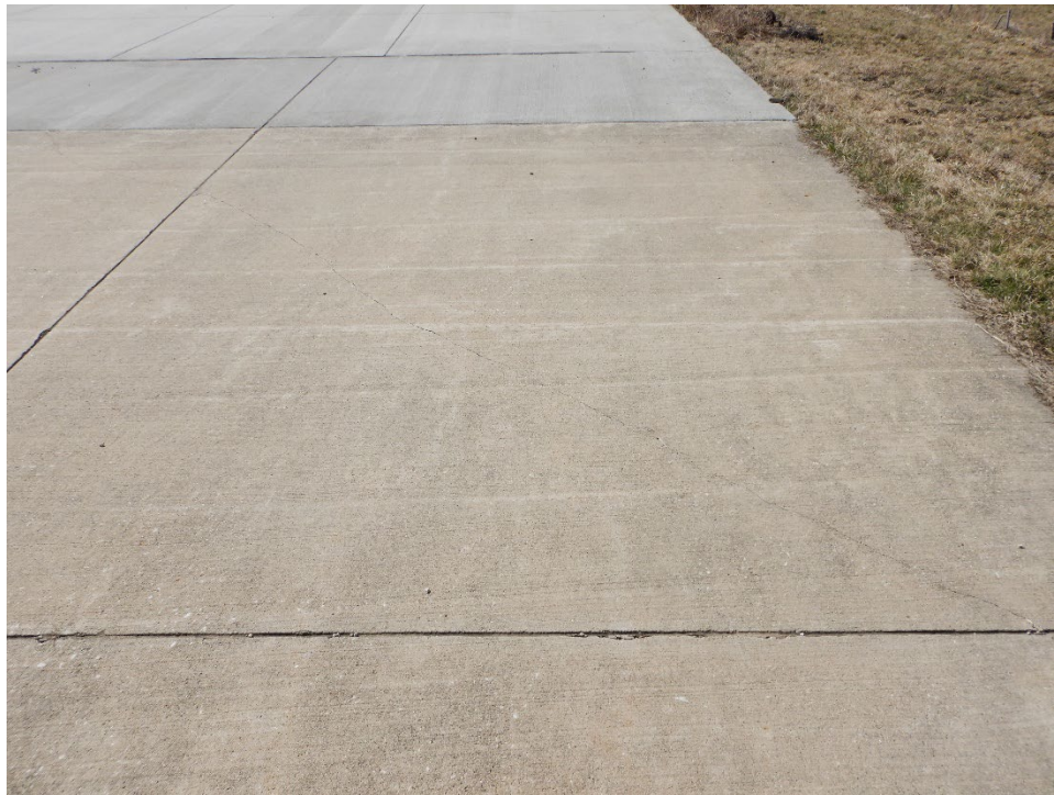
TH01SC-01. LTD Cracking (Sample Unit No. 02).
