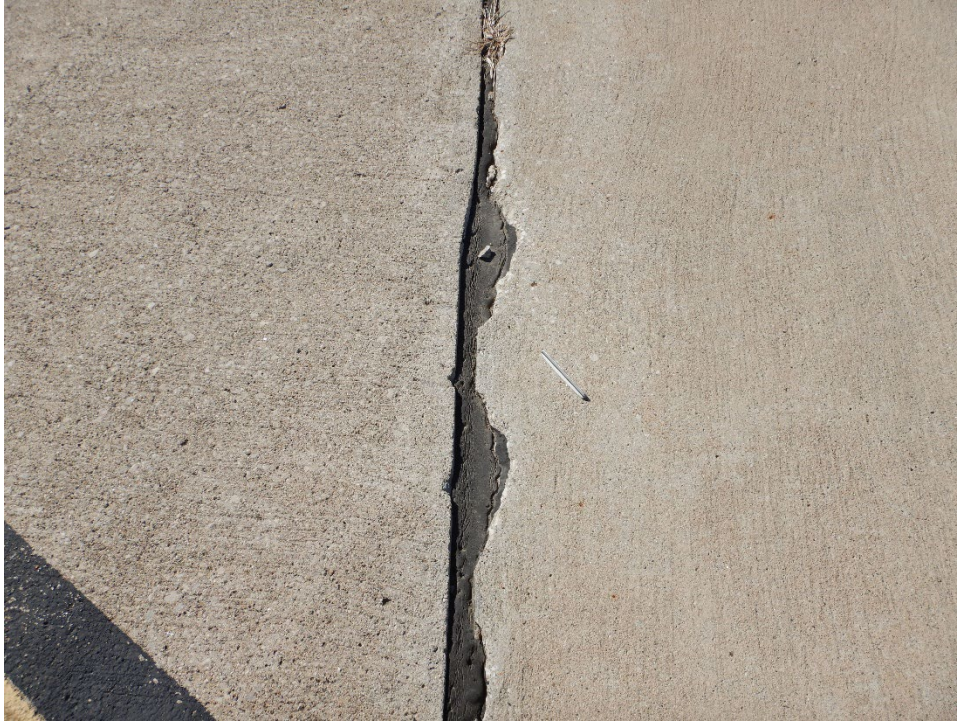
T01SC-02. Joint Spalling (Sample Unit No. 02).
