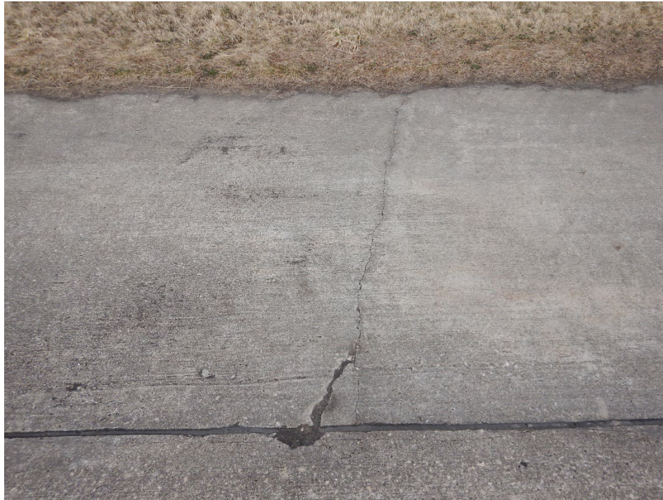
R18SC-05. LTD Cracking (Sample Unit No. 05).
