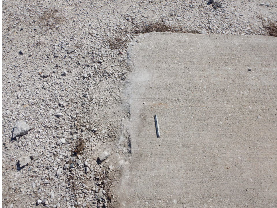
TH01SC-01. Joint Spalling (Sample Unit No. 06).
