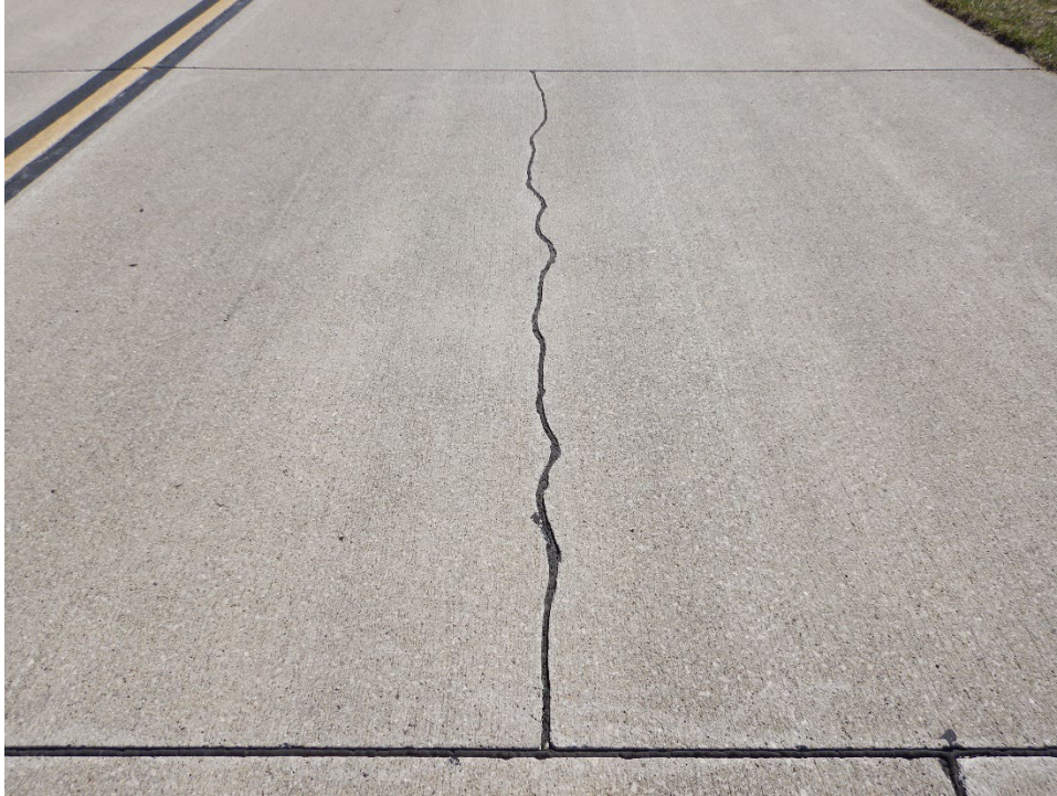
T01SC-01. LTD Cracking (Sample Unit No. 02).
