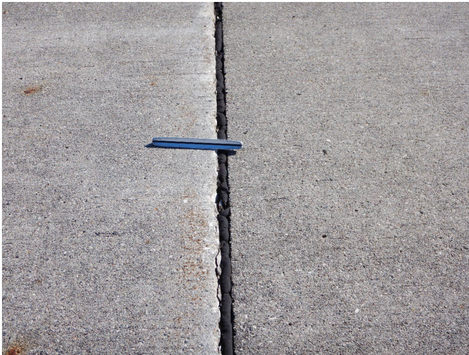
R14SC-01. Faulting (Sample Unit No. 25).
