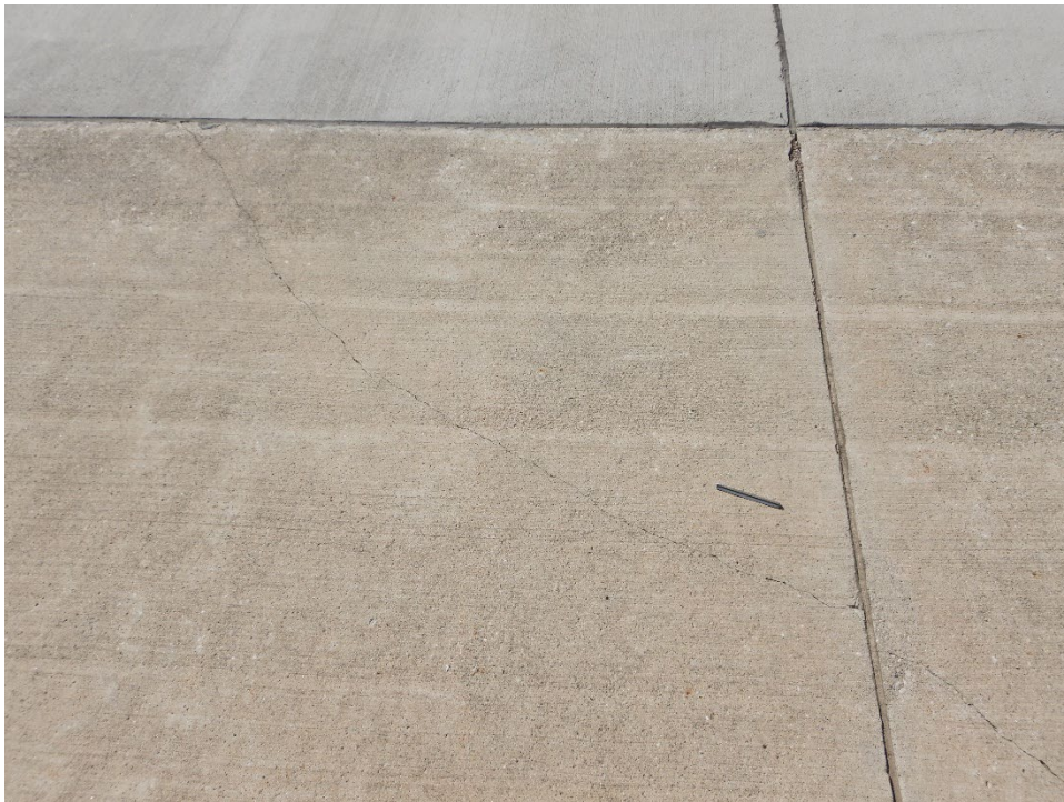
TH01SC-01. Corner Break (Sample Unit No. 02).
