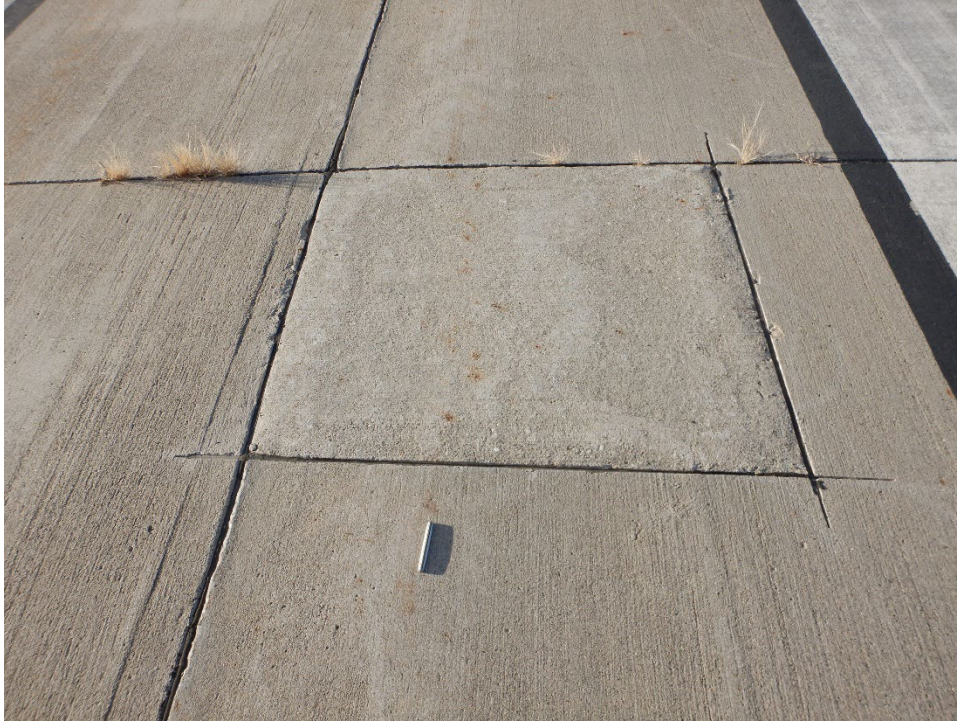
R18SC-04. Large Patching (Sample Unit No. 09).
