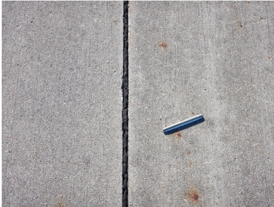
R14SC-01. Joint Seal Damage (Sample Unit No. 07).
