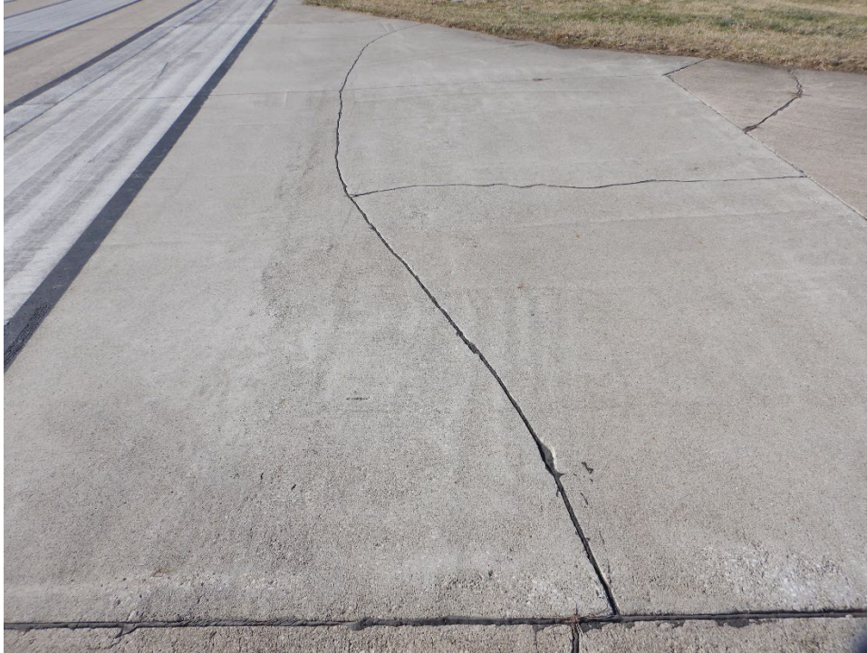
R18SC-06. LTD Cracking (Sample Unit No. 01).
