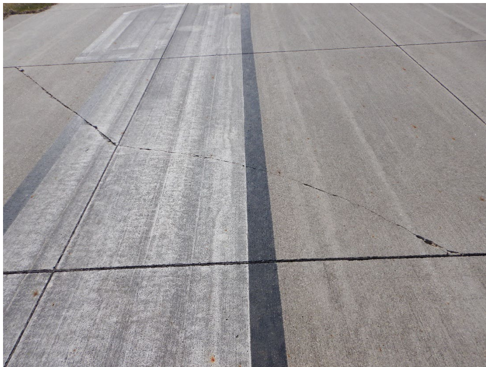
R14SC-01. LTD Cracking (Sample Unit No. 02).
