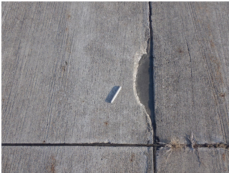
R18SC-04. Joint Spalling (Sample Unit No. 08).
