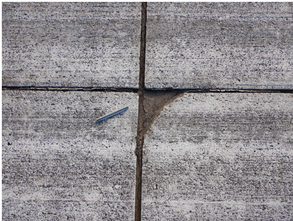
R18SC-01. Corner Spalling (Sample Unit No. 02).
