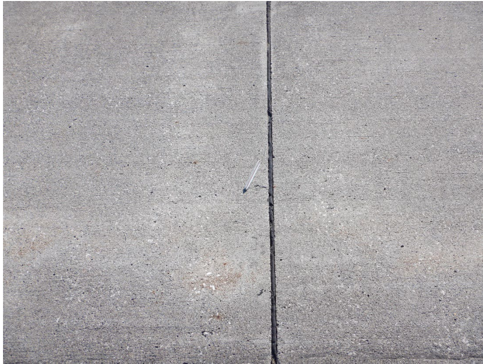
R18SC-02. Joint Seal Damage (Sample Unit No. 02).
