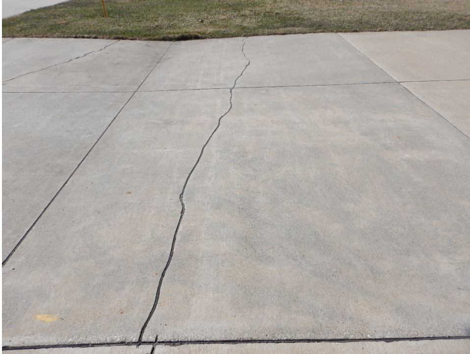
A01SC-01. LTD Cracking (Additional Sample Unit No. 08).
