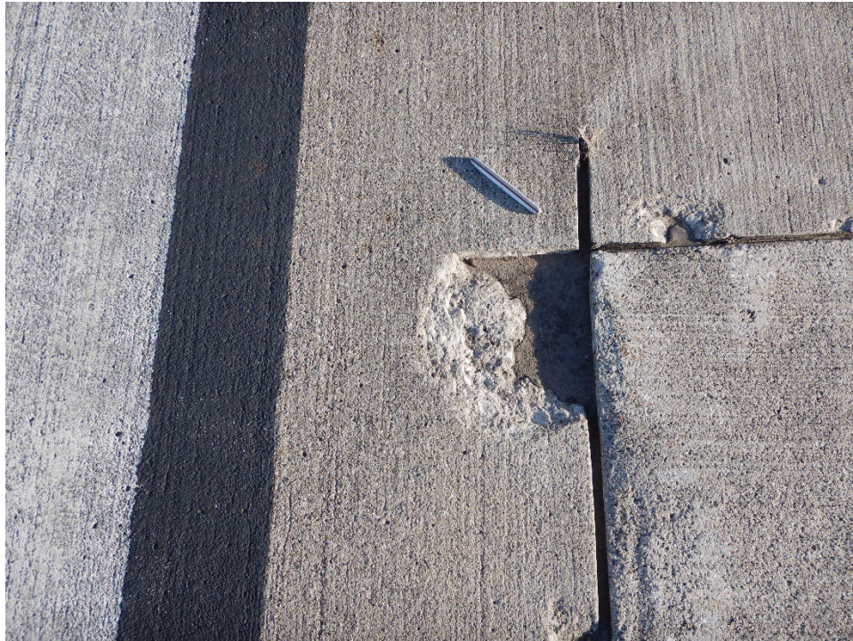
R18SC-04. Corner Spalling (Sample Unit No. 08).
