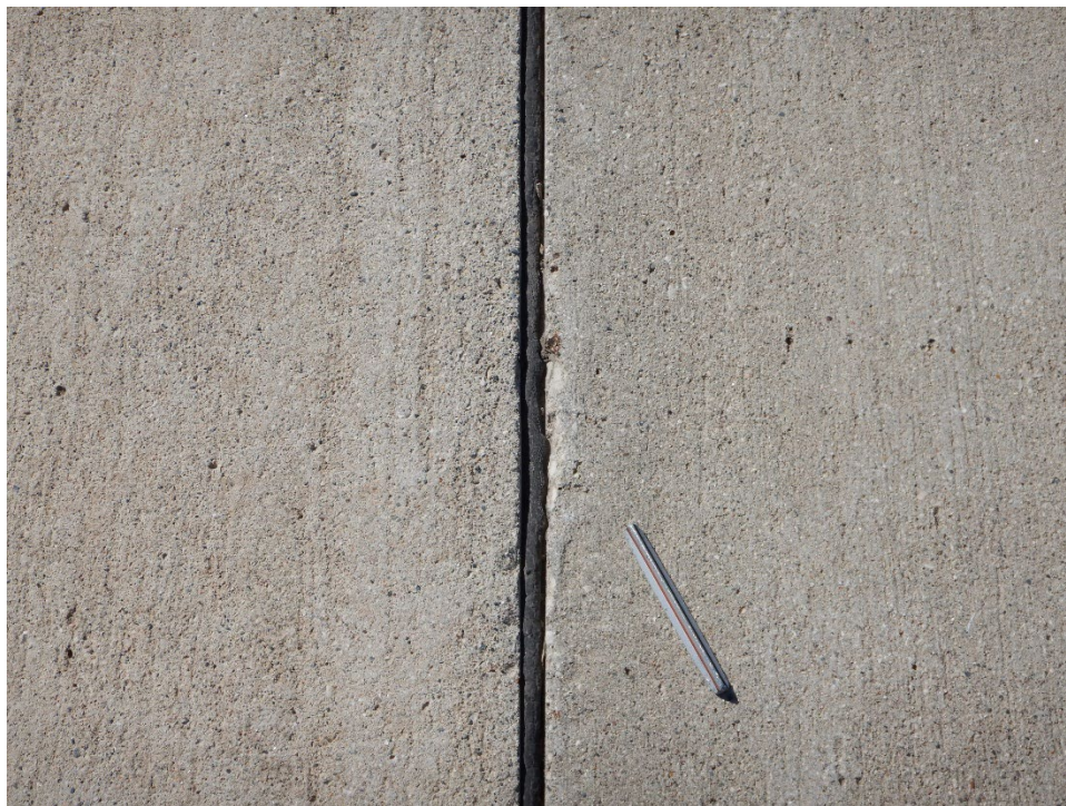
A01SC-01. Joint Seal Damage (Sample Unit No. 07).
