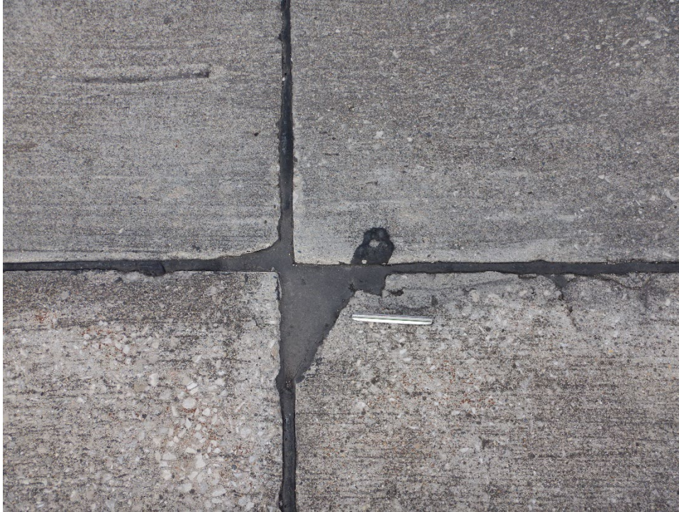
R18SC-01. Corner Spalling (Sample Unit No. 42).
