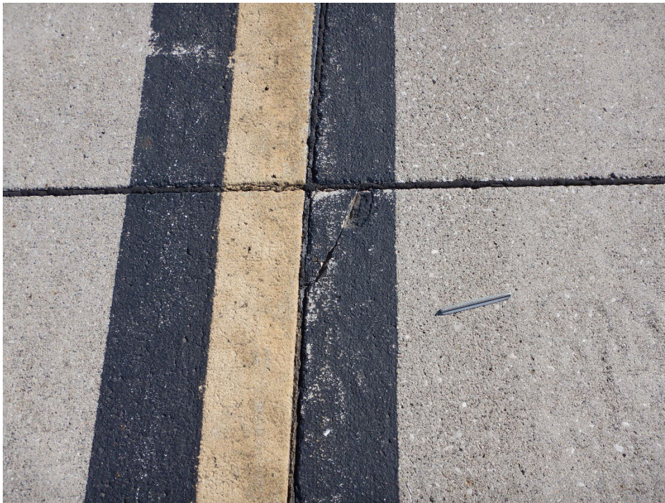
T02SC-01. Corner Spalling (Sample Unit No. 02).
