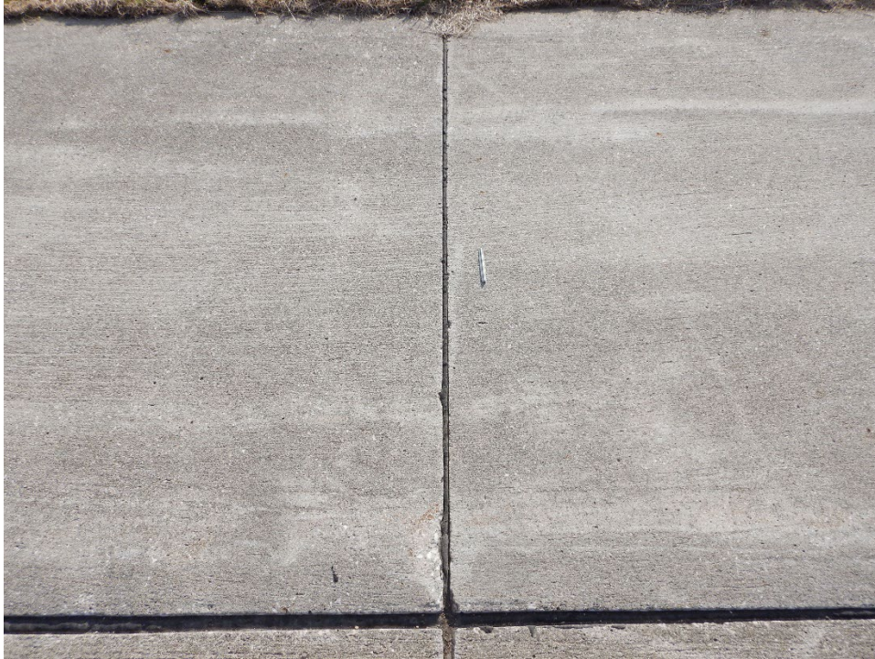
R18SC-03. Joint Seal Damage (Sample Unit No. 01).
