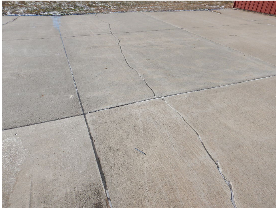
A01SC-01. LTD Cracking (Additional Sample Unit No. 08).
