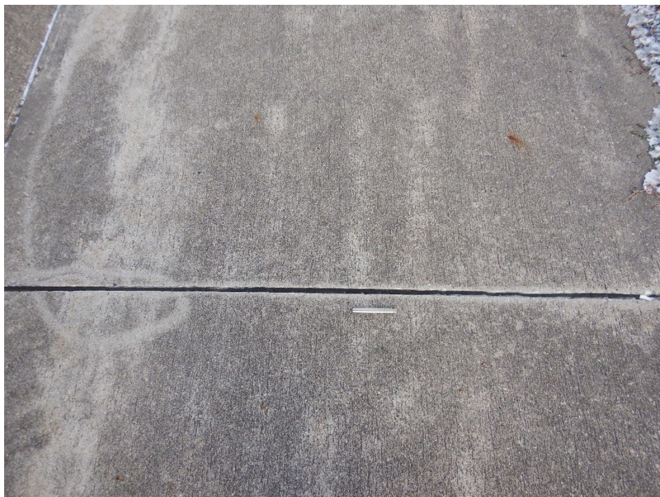
R18SC-02. Joint Seal Damage (Sample Unit No. 03).
