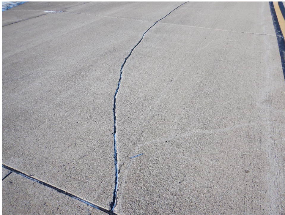
T01SC-01. LTD Cracking (Sample Unit No. 01).
