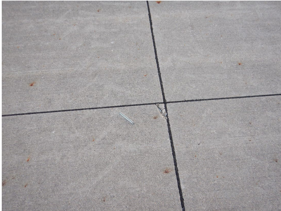
R14SC-01. Corner Spalling (Sample Unit No. 20).
