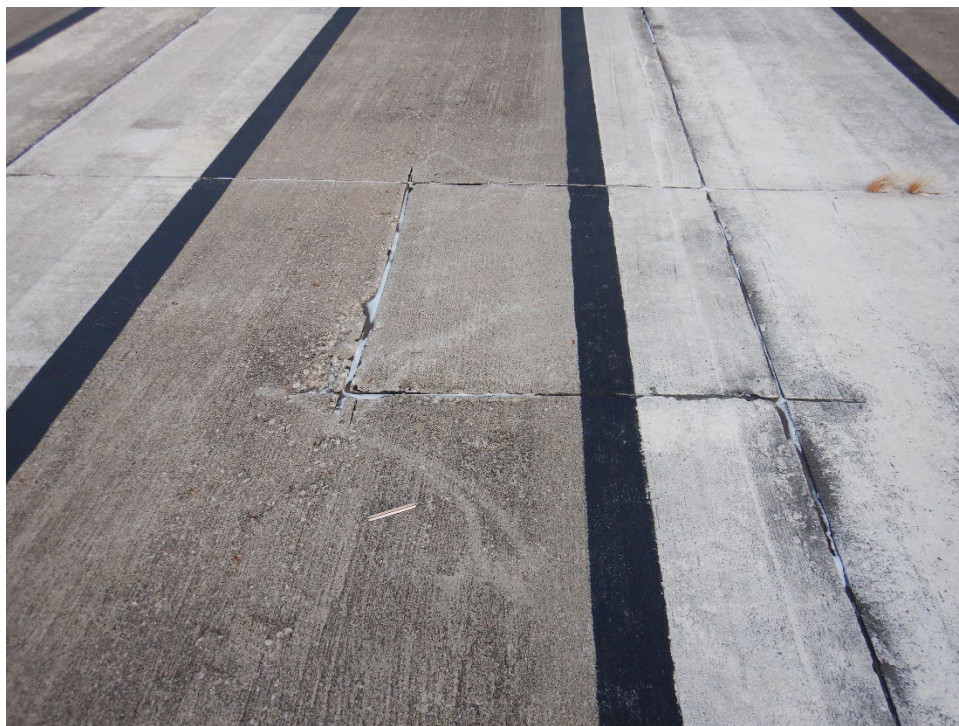
R18SC-04. Large Patching (Sample Unit No. 10).
