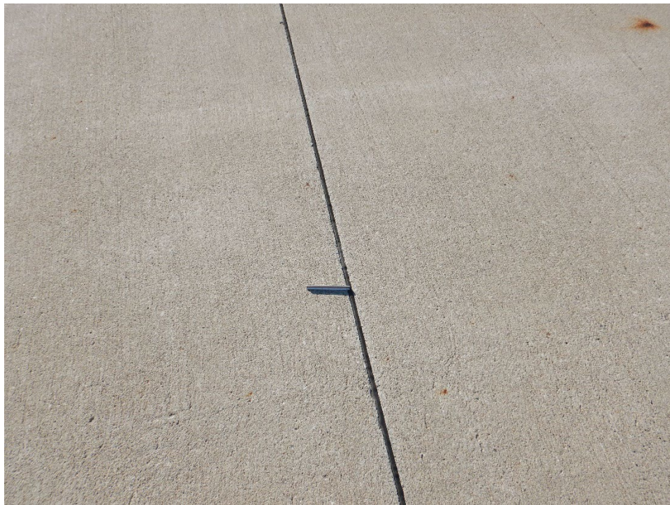
A01SC-01. Joint Seal Damage (Sample Unit No. 01).
