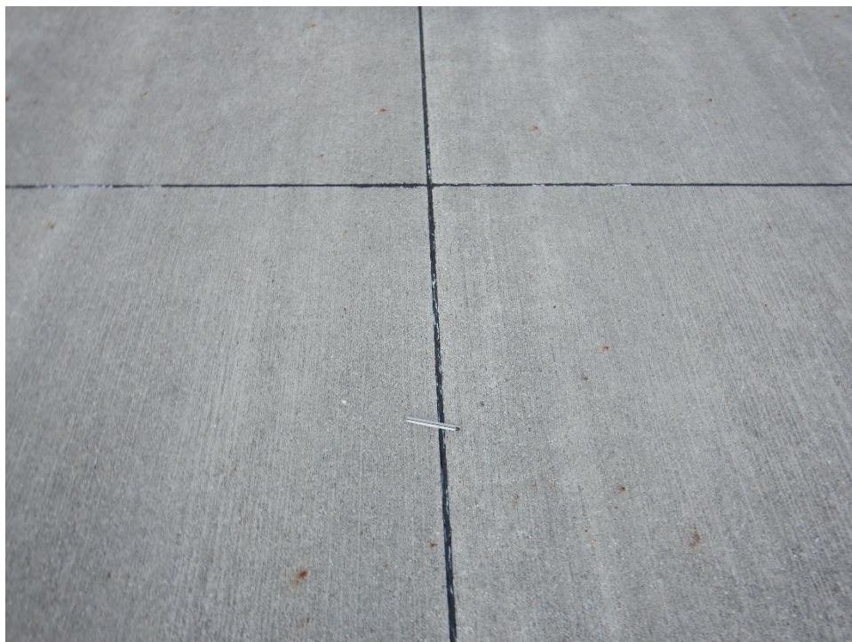
R14SC-01. Joint Seal Damage (Sample Unit No. 11).
