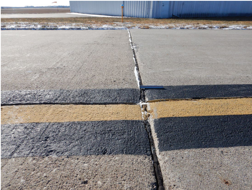
T02SC-01. Faulting (Sample Unit No. 01).
