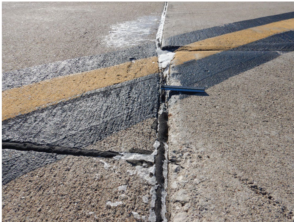
T01SC-02. Faulting (Sample Unit No. 02).
