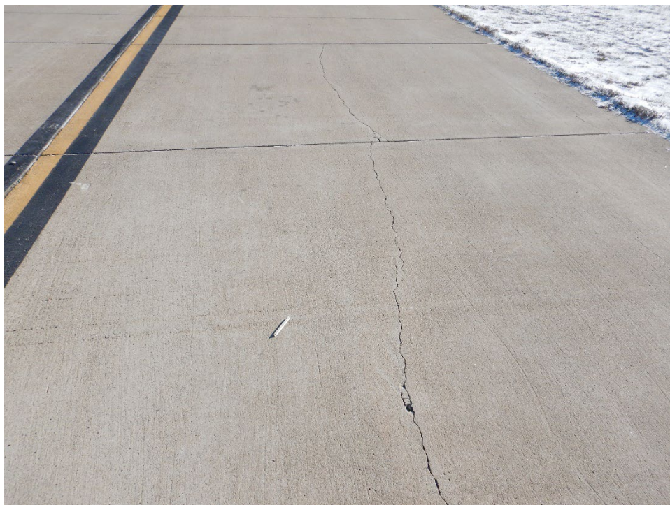
TH01SC-01. LTD Cracking (Sample Unit No. 01).
