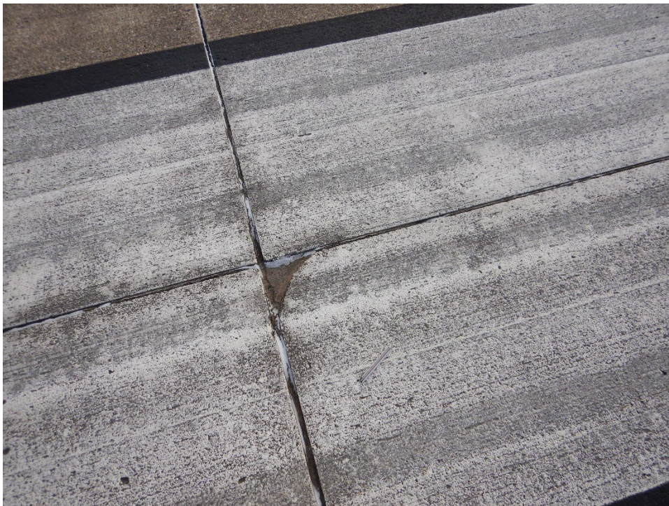
R18SC-01. Corner Spalling (Sample Unit No. 02).
