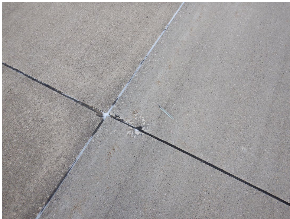
R18SC-03. Joint Spalling (Sample Unit No. 05).
