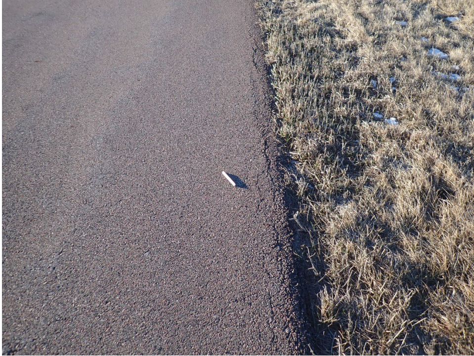
R16RR-02. Alligator Cracking (Sample Unit No. 17).
