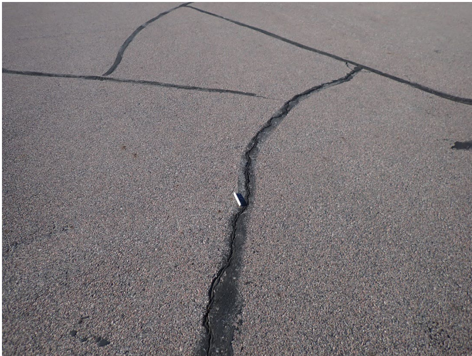
A01RR-01. L&T Cracking (Sample Unit No. 03).
