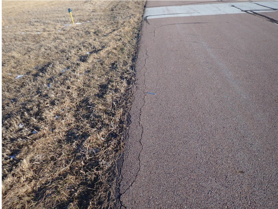
R16RR-03. Alligator Cracking (Sample Unit No. 01).
