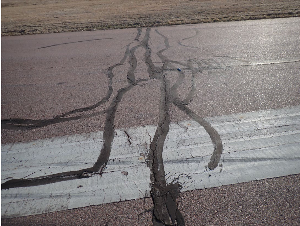
R16RR-03. L&T Cracking (Sample Unit No. 02).
