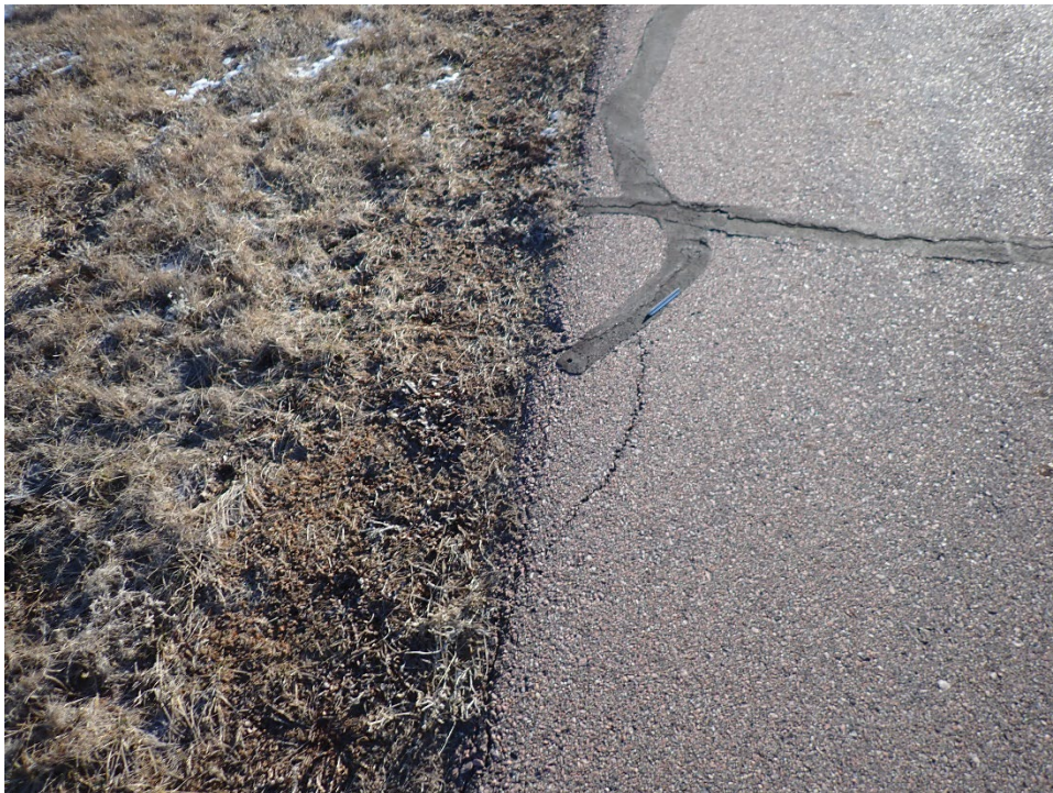
T01RR-01. Alligator Cracking (Sample Unit No. 01).
