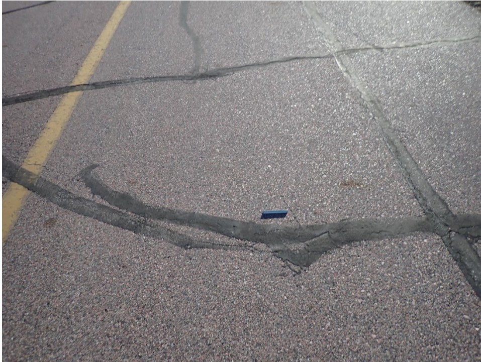
T01RR-01. L&T Cracking (Sample Unit No. 01).
