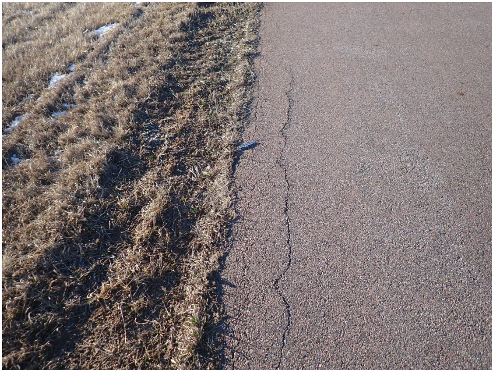
R16RR-02. Alligator Cracking (Sample Unit No. 21).
