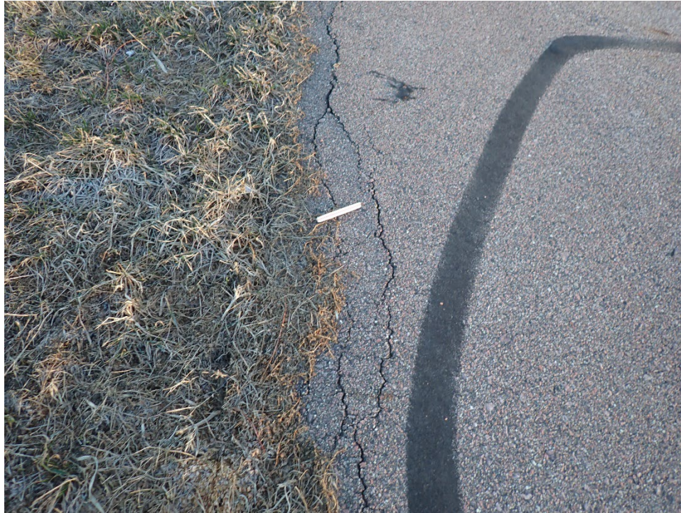
R16RR-01. Alligator Cracking (Sample Unit No. 03).
