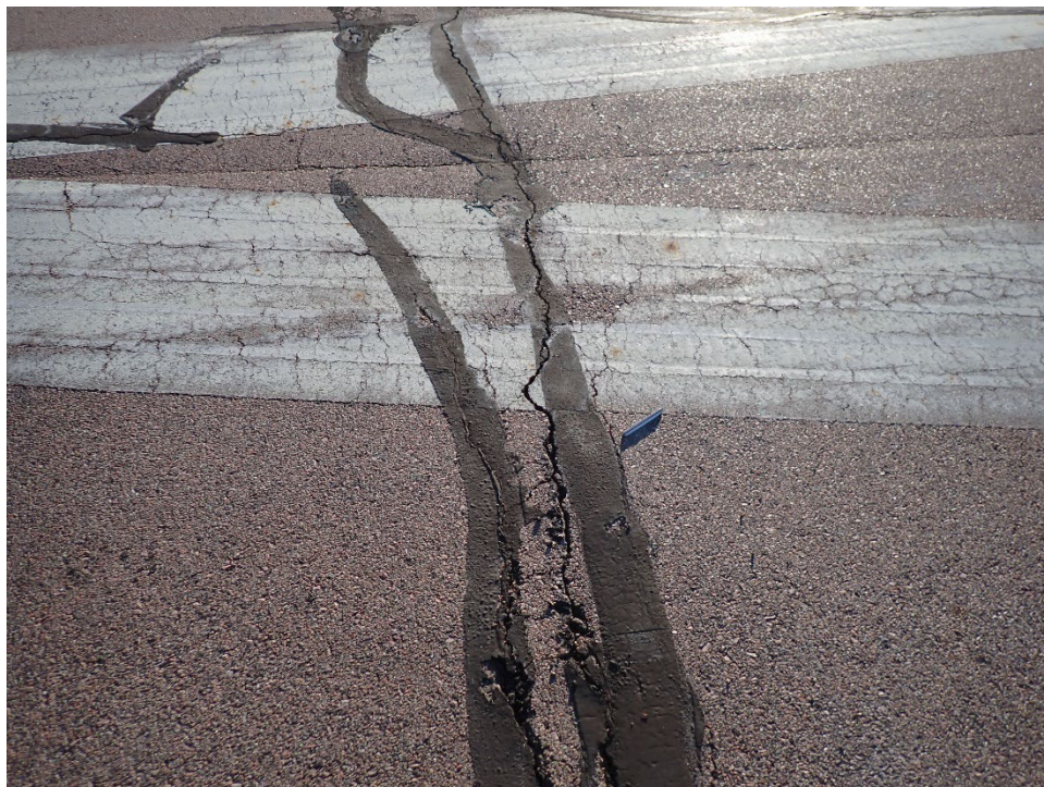
R16RR-03. L&T Cracking (Sample Unit No. 01).
