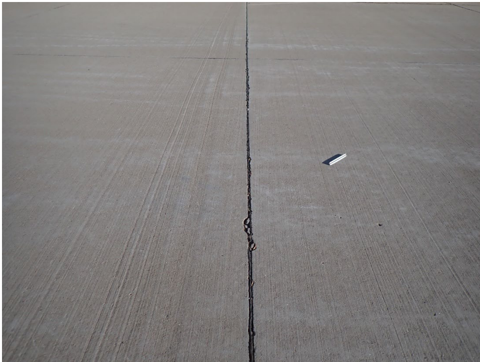
A01RR-02. Joint Seal Damage (Sample Unit No. 02).
