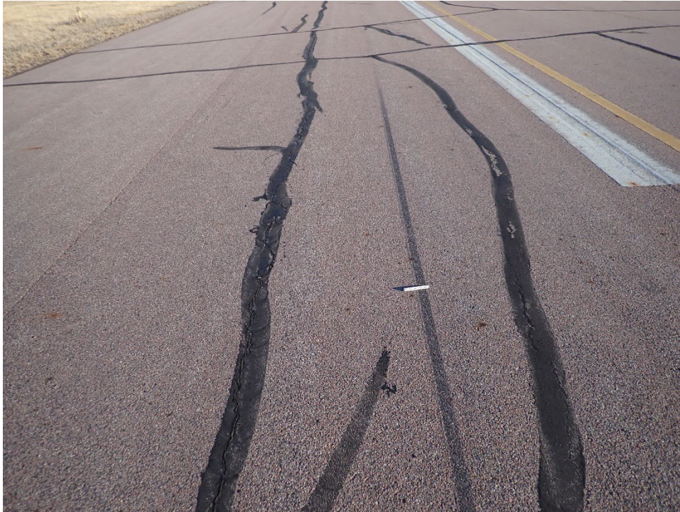
R16RR-02. L&T Cracking (Sample Unit No. 17).
