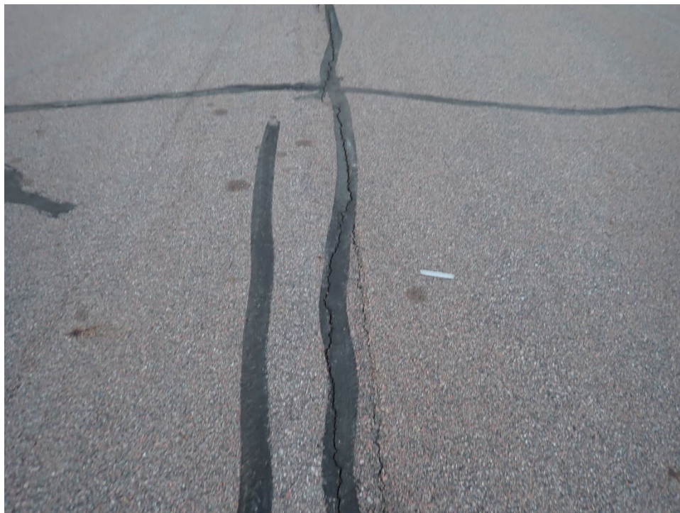
R16RR-01. L&T Cracking (Sample Unit No. 01).
