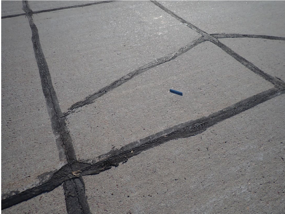
A01RR-03. LTD Cracking (Sample Unit No. 05).
