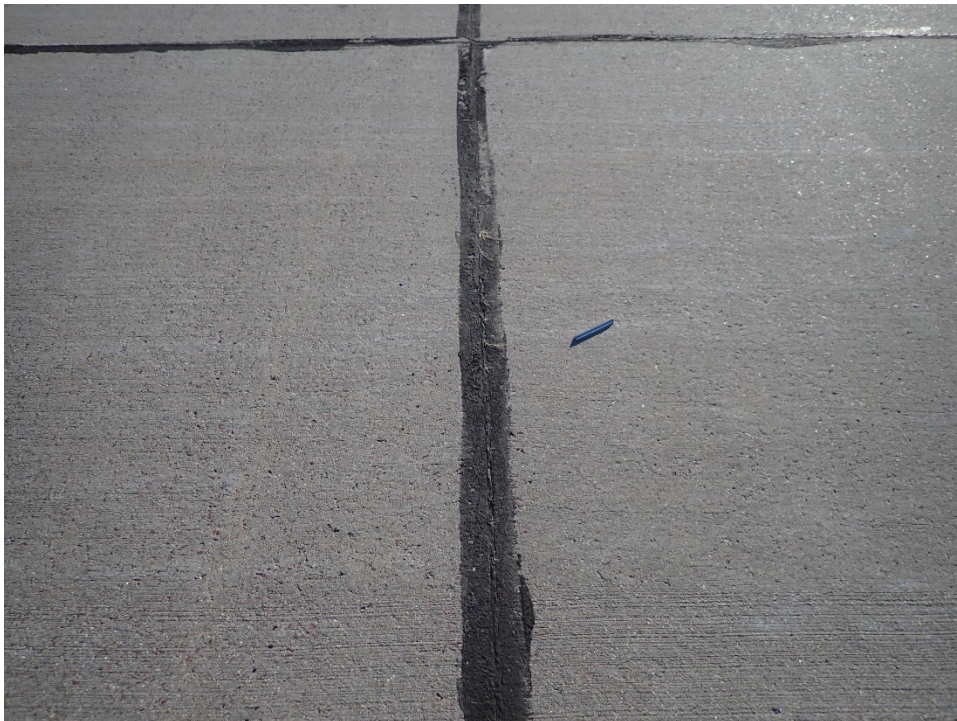
A01RR-03. Joint Seal Damage (Sample Unit No. 05).
