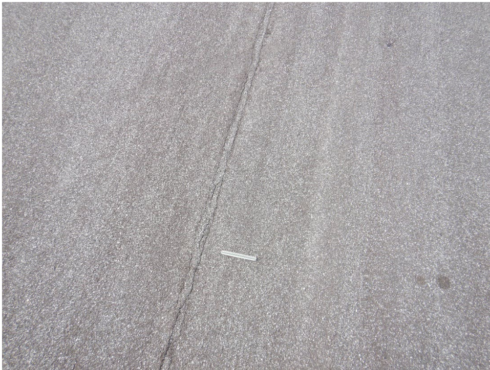
R12PO-02. Joint Reflection Cracking (Sample Unit No. 08).
