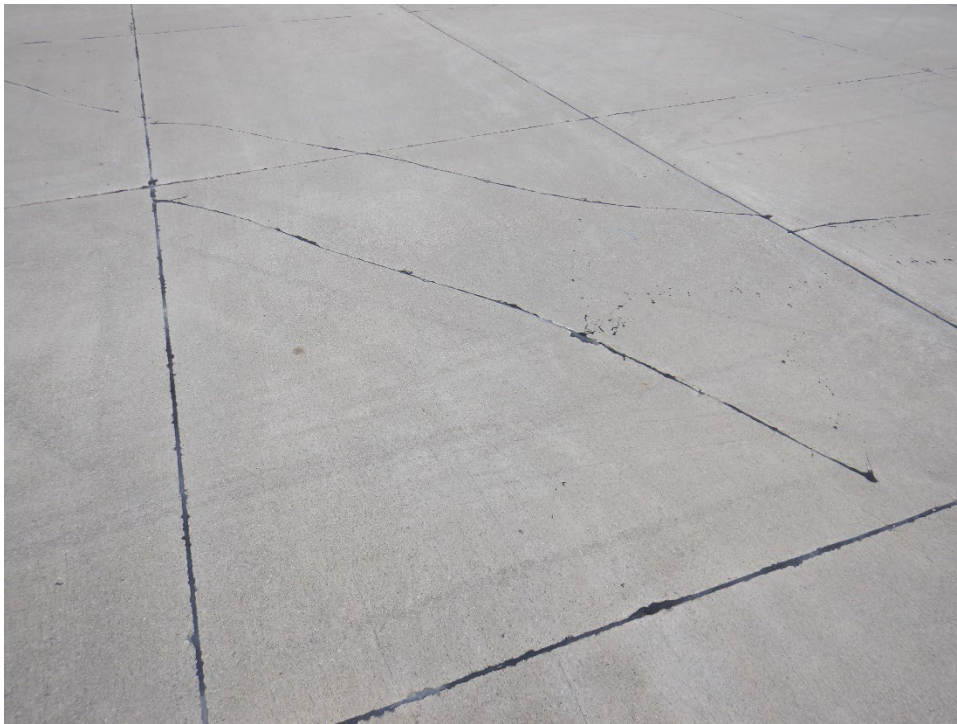
A01PO-01. LTD Cracking (Sample Unit No. 03).
