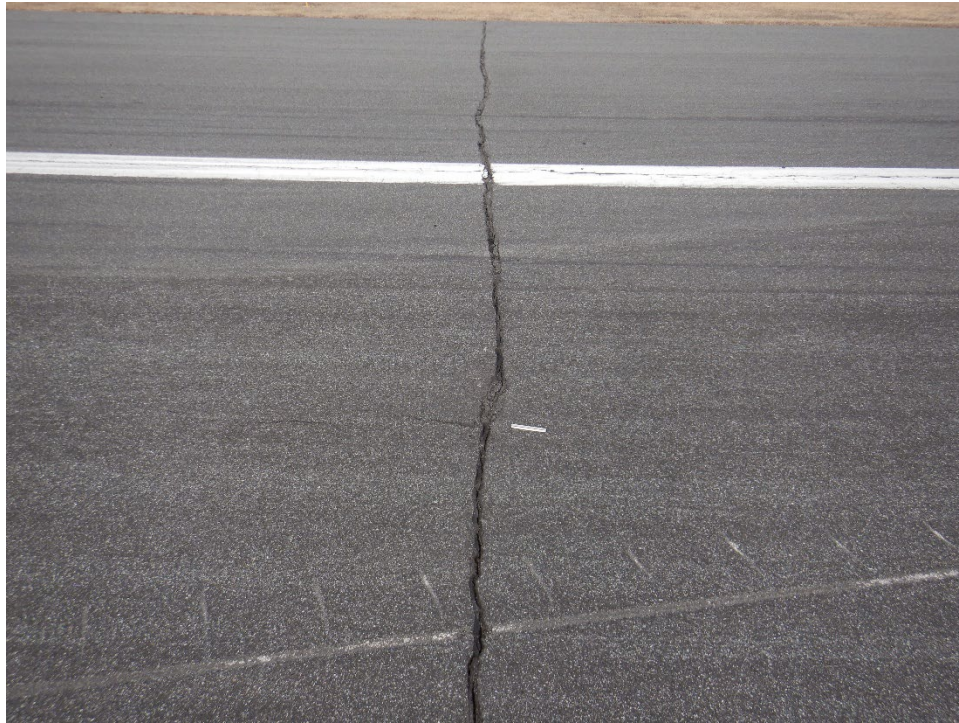
R12PO-01. Joint Reflection Cracking (Sample Unit No. 28).
