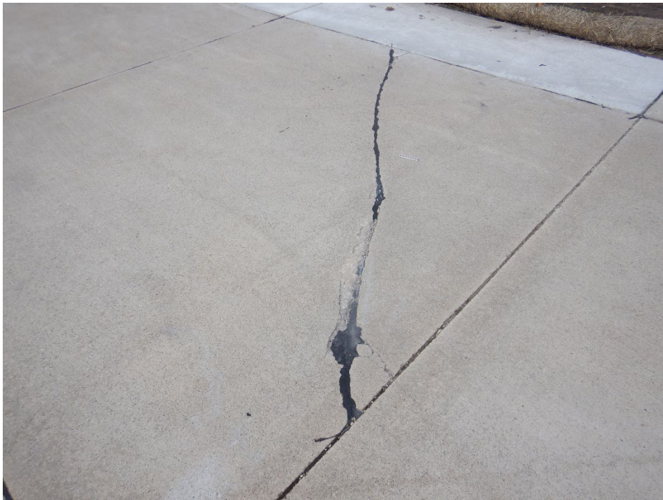
T01PO-02. LTD Cracking (Sample Unit No. 02).
