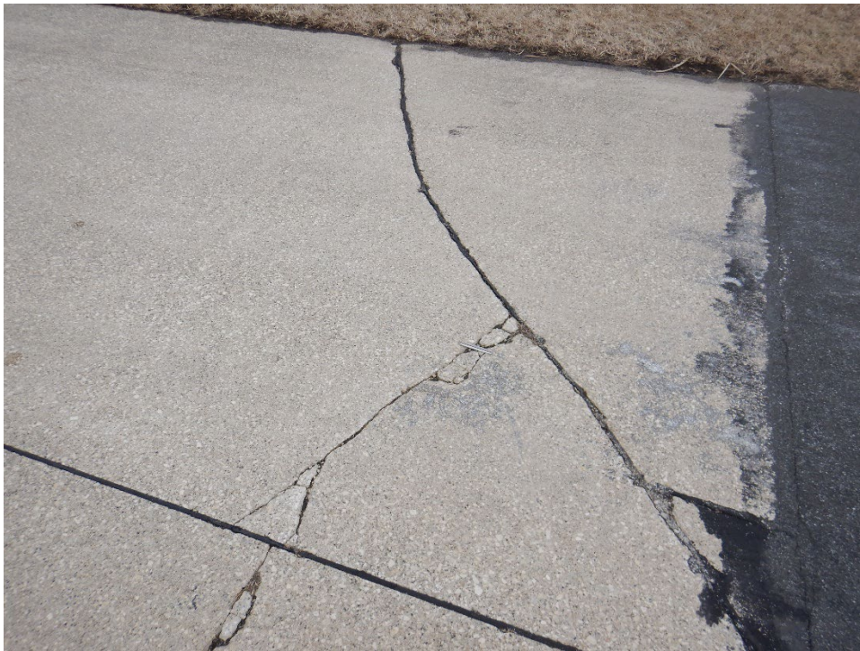
T01PO-01. LTD Cracking (Sample Unit No. 01).
