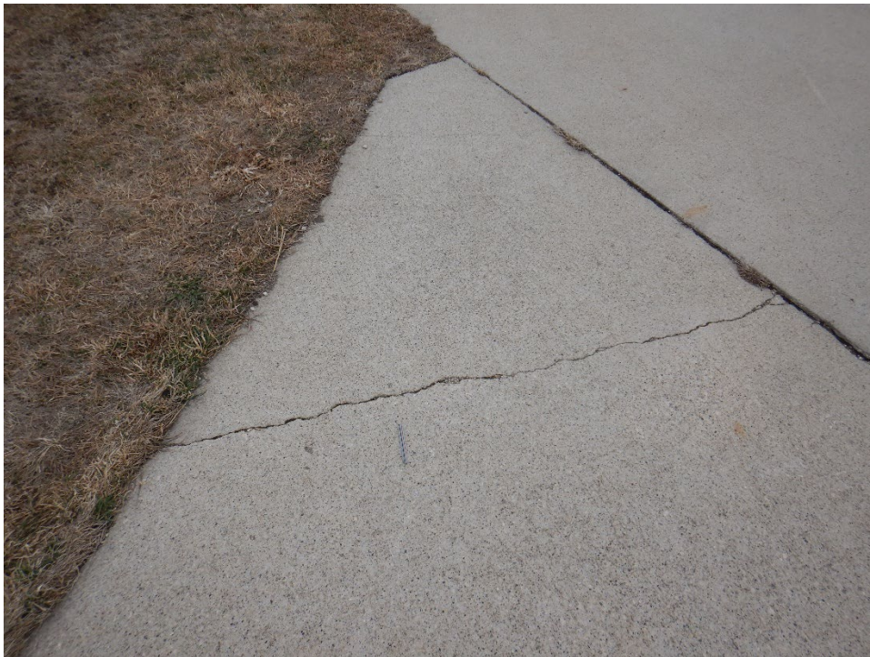
TH01PO-02. LTD Cracking (Sample Unit No. 01).
