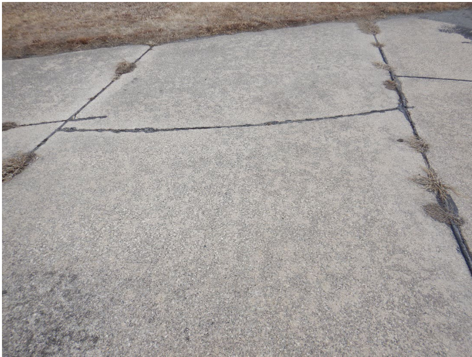
R12PO-04. LTD Cracking (Sample Unit No. 01).
