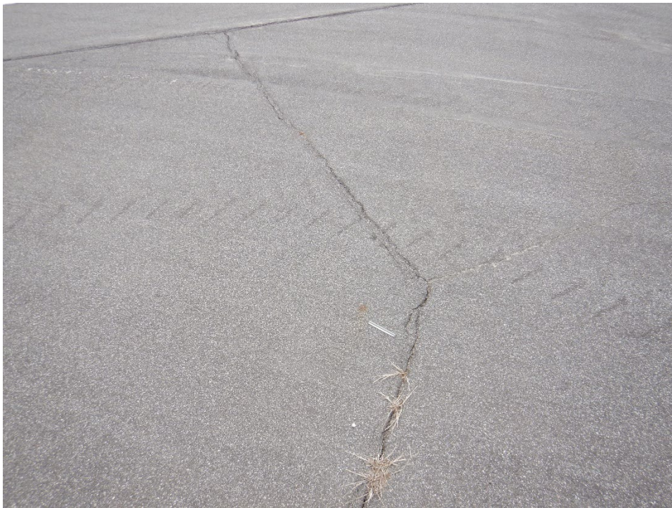
T02PO-03. Joint Reflection Cracking (Sample Unit No. 01).
