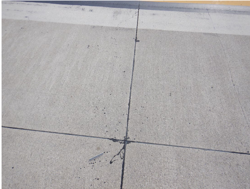
T02PO-02. Joint Seal Damage (Sample Unit No. 03).
