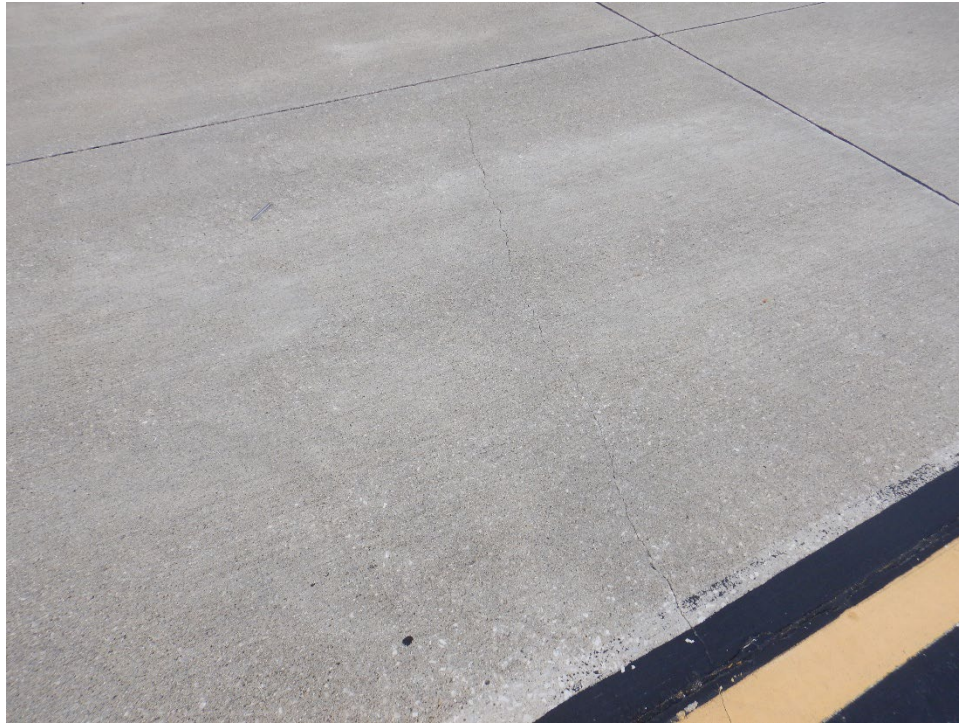
T02PO-01. LTD Cracking (Sample Unit No. 01).
