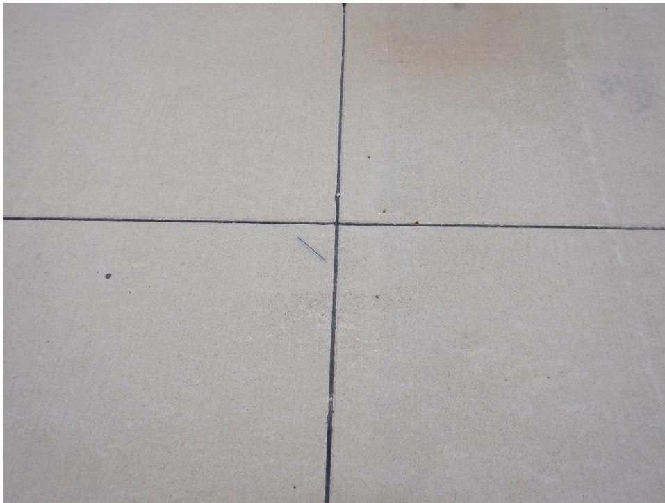
TH01PO-04. Joint Seal Damage (Sample Unit No. 05).
