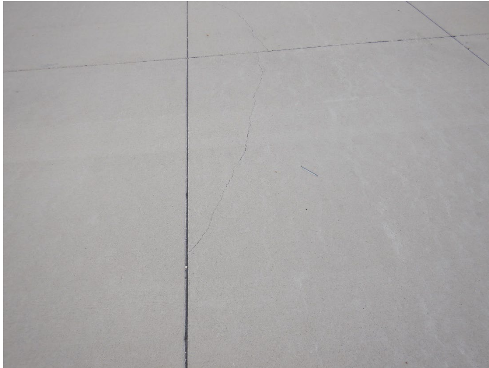
TH01PO-04. LTD Cracking (Sample Unit No. 05).
