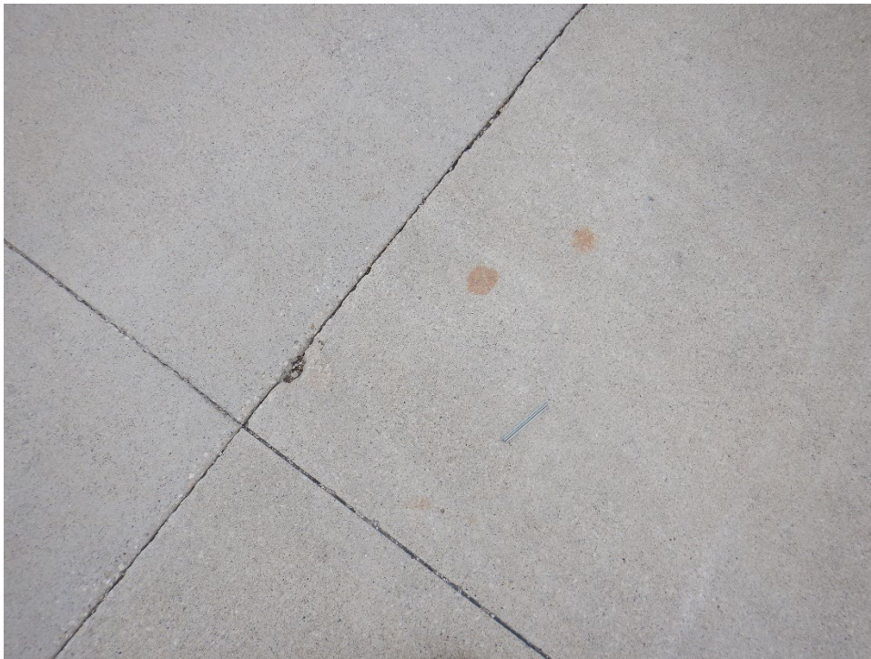
TH01PO-01. Joint Seal Damage (Sample Unit No. 01).
