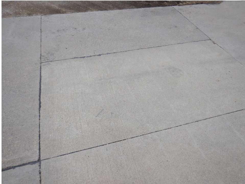
TH01PO-01. Large Patching (Sample Unit No. 01).
