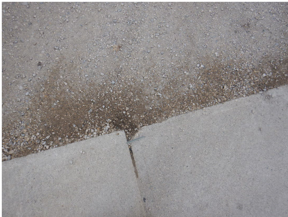
TH01PO-03. Corner Spalling (Sample Unit No. 01).
