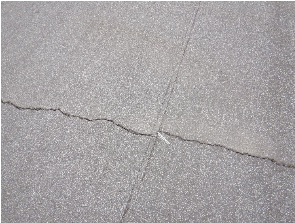
R12PO-03. Joint Reflection Cracking (Sample Unit No. 02).
