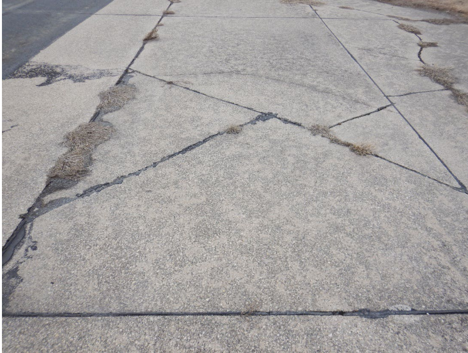
R12PO-04. Shattered Slab (Sample Unit No. 01).
