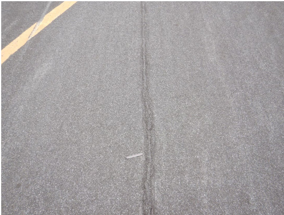
T01PO-03. Joint Reflection Cracking (Sample Unit No. 01).
