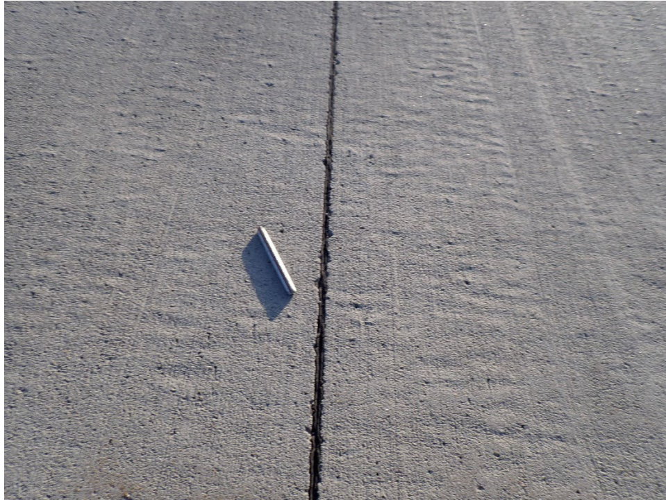
A01PE-05. Joint Seal Damage (Sample Unit No. 01).
