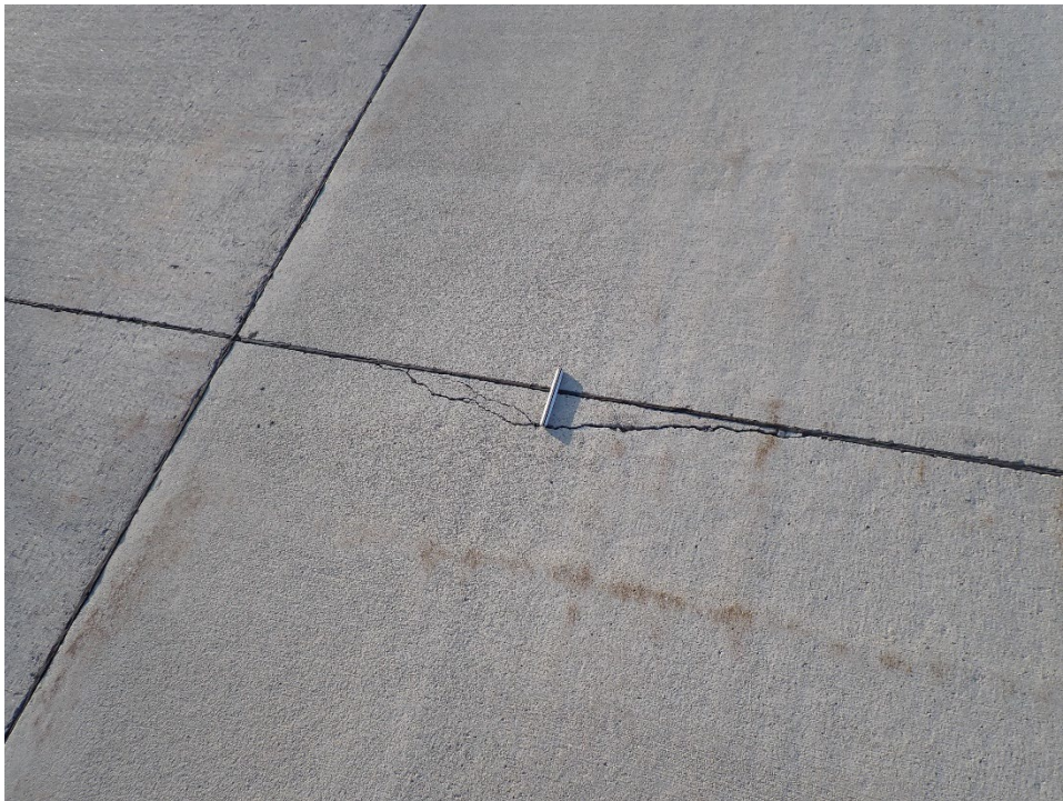
A01PE-03. Joint Spalling (Sample Unit No. 03).
