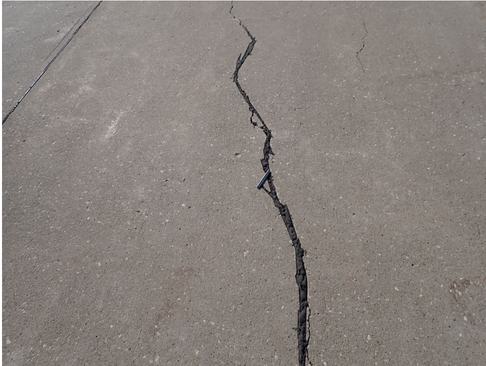
R16PE-03. LTD Cracking (Sample Unit No. 31).
