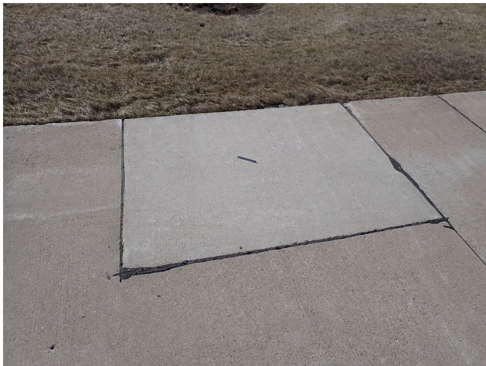
R16PE-07. Large Patching (Sample Unit No. 04).
