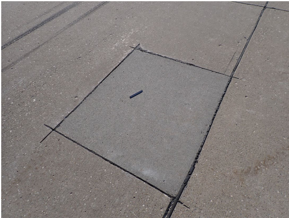
R16PE-03. Large Patching (Sample Unit No. 31).
