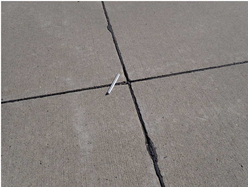
R16PE-08. Joint Seal Damage (Sample Unit No. 01).
