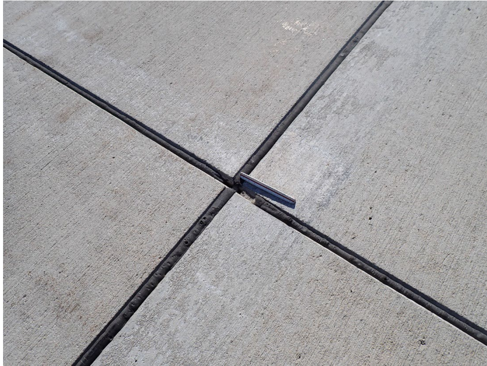
R16PE-01. Joint Seal Damage (Sample Unit No. 12).
