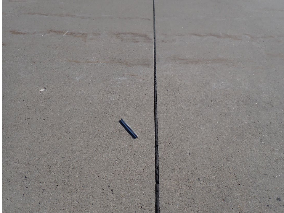
R16PE-10. Joint Seal Damage (Sample Unit No. 02).
