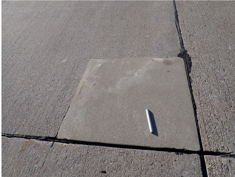
R16PE-06. Large Patching (Sample Unit No. 20).
