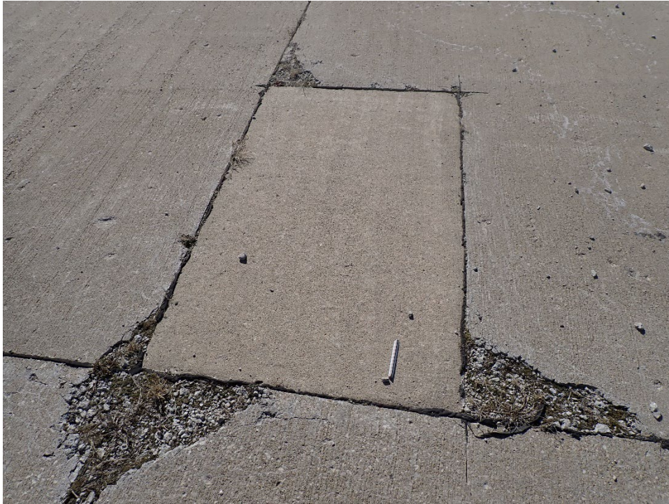
R16PE-11. Large Patching (Sample Unit No. 03).
