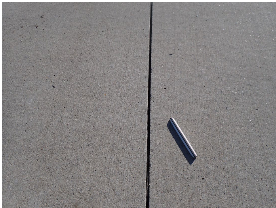
TH01PE-02. Joint Seal Damage (Sample Unit No. 01).
