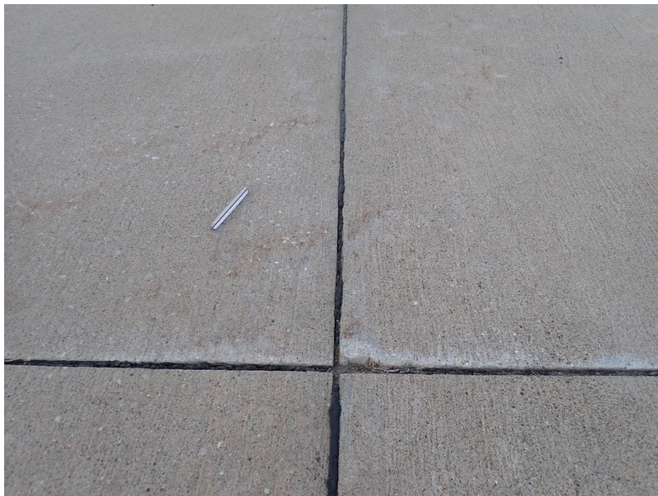
A01PE-04. Joint Seal Damage (Sample Unit No. 02).
