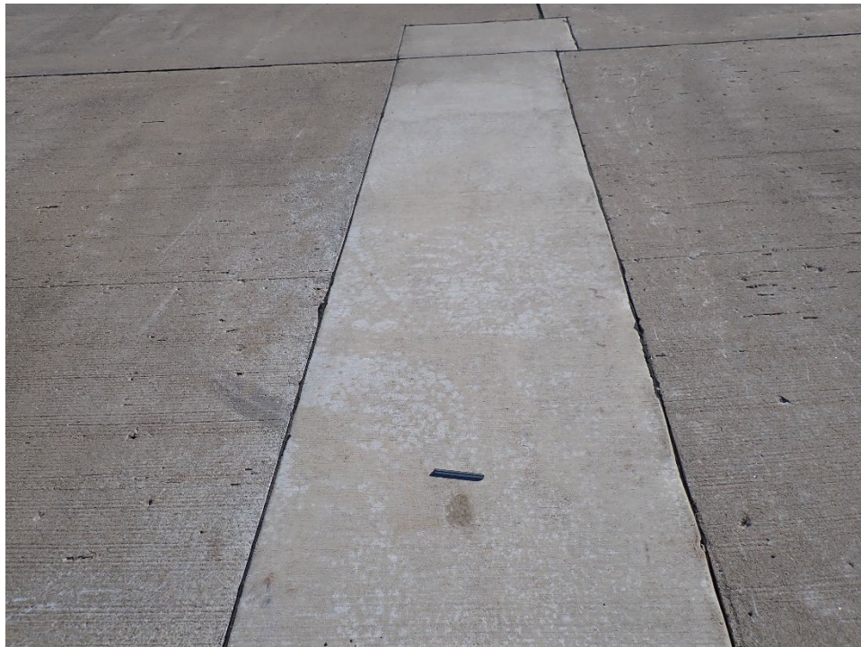
R16PE-05. Large Patching (Sample Unit No. 01).
