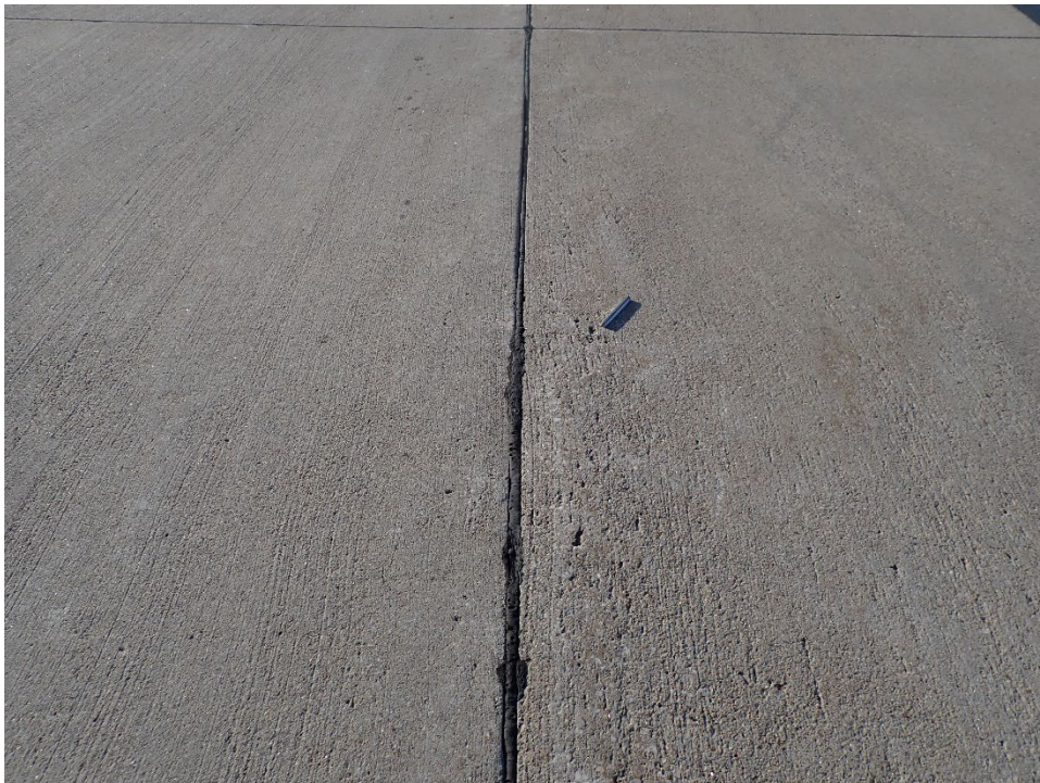
R16PE-06. Joint Seal Damage (Sample Unit No. 20).
