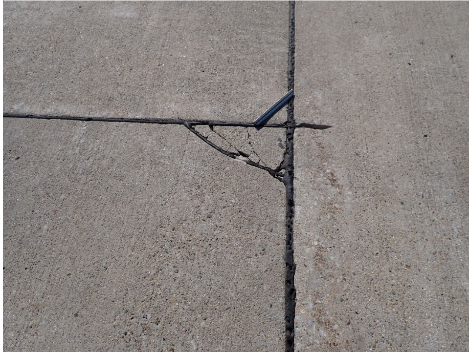
R16PE-07. Corner Spalling (Sample Unit No. 04).
