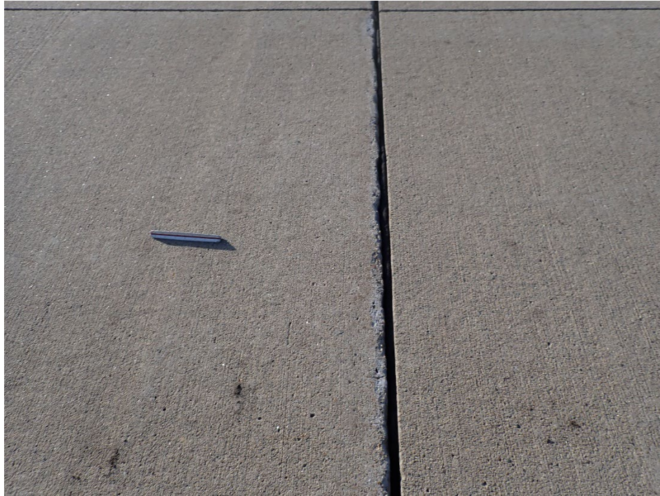
R16PE-09. Joint Seal Damage (Sample Unit No. 05).
