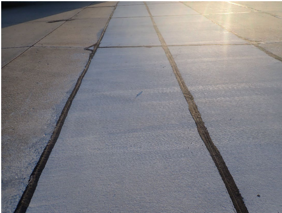
A01PE-02. Large Patching (Sample Unit No. 01).
