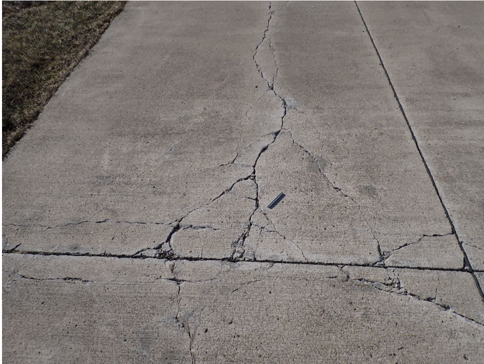
TH01PE-01. Shattered Slab (Sample Unit No. 06).
