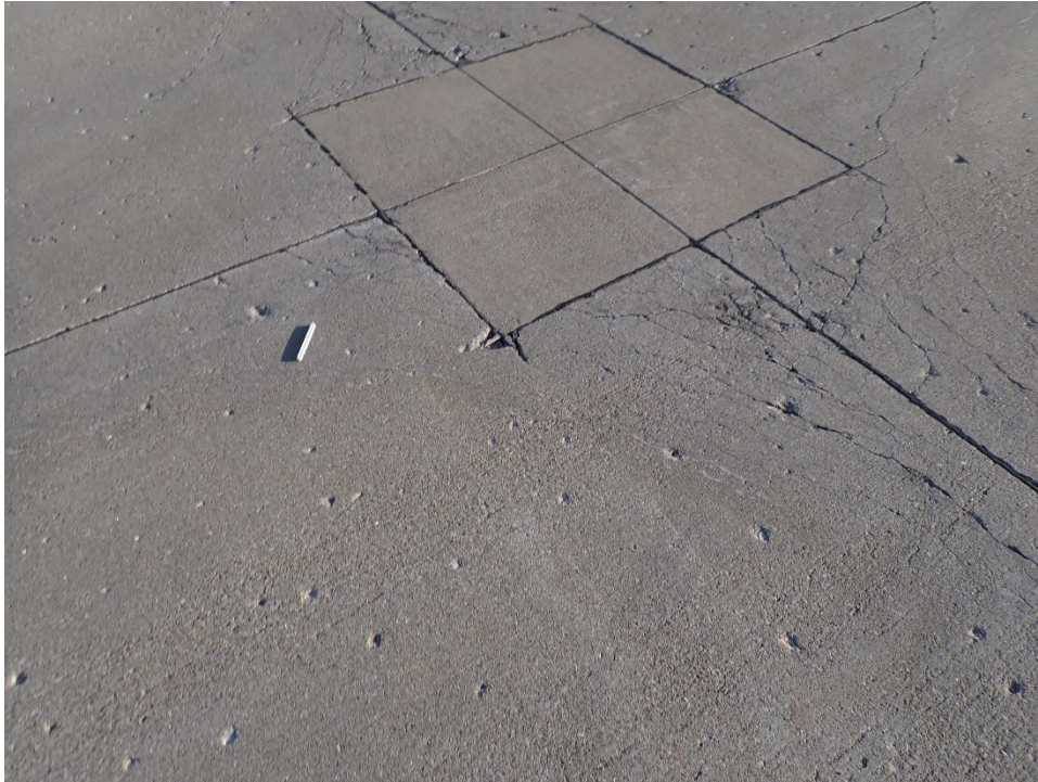
A01PE-01. Small Patching (Sample Unit No. 09).
