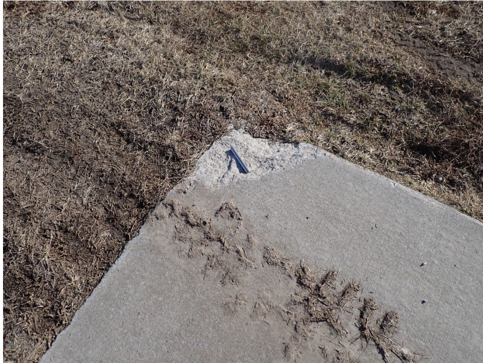
TH01PE-02. Corner Spalling (Sample Unit No. 02).
