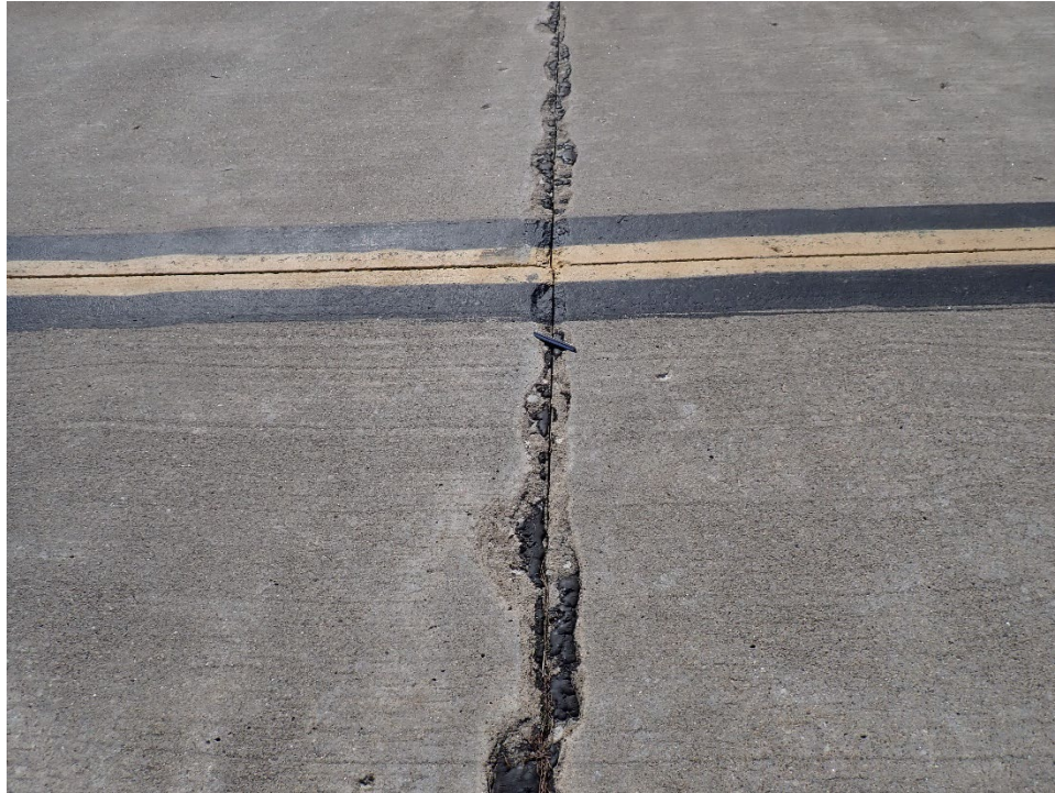
TH01PE-01. Joint Seal Damage (Sample Unit No. 01).
