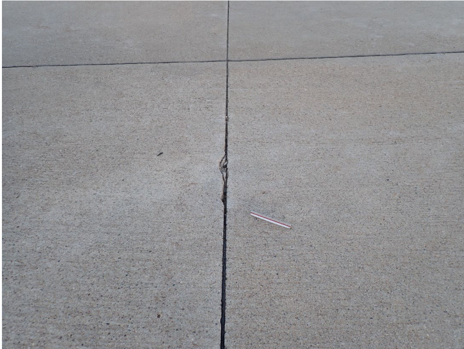
A01PE-03. Joint Seal Damage (Sample Unit No. 03).
