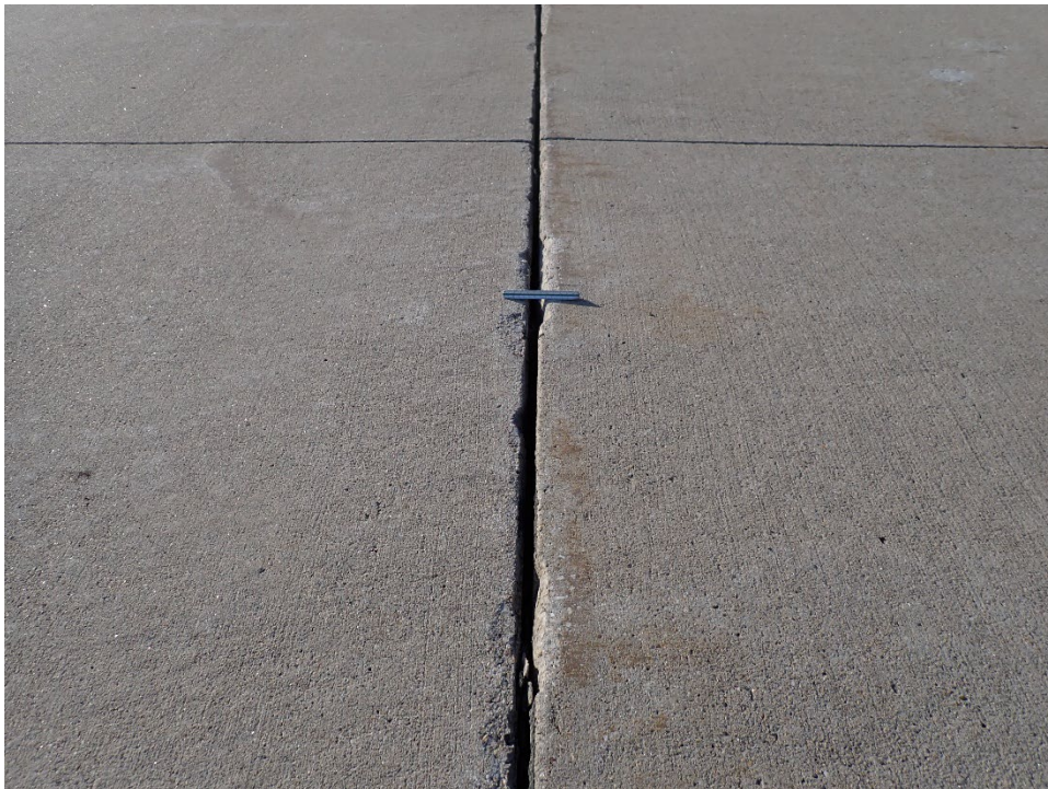
R16PE-09. Faulting (Sample Unit No. 05).
