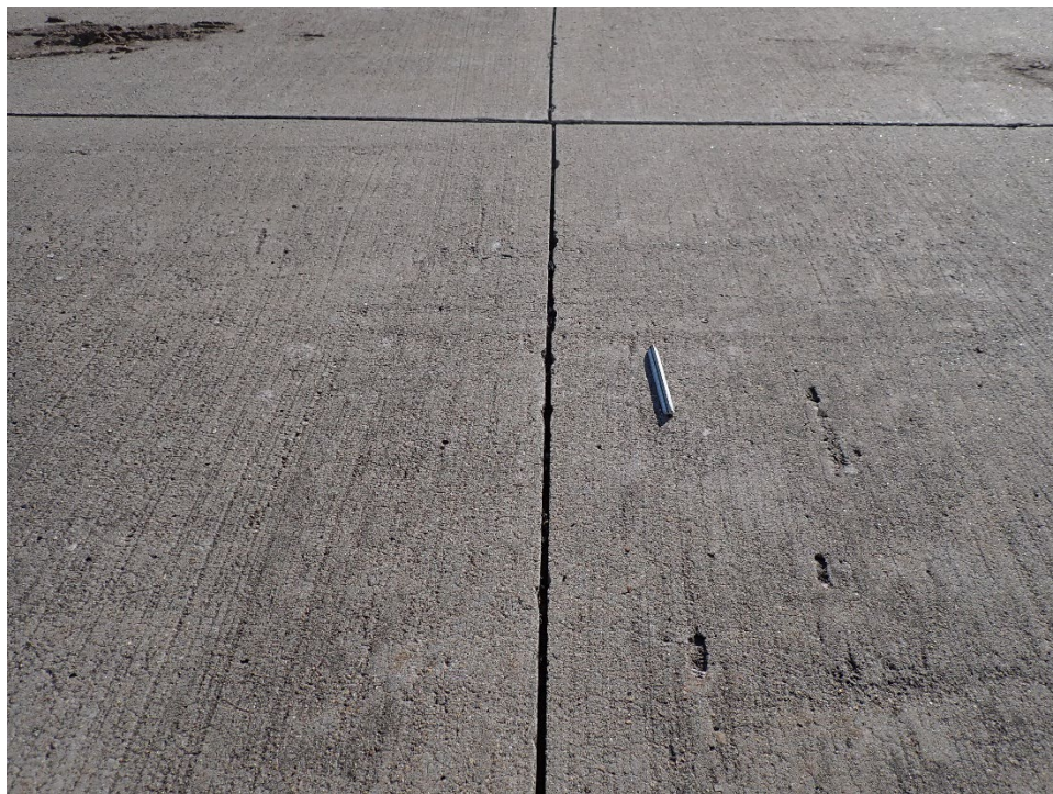
TH01PE-01. Joint Seal Damage (Sample Unit No. 05).
