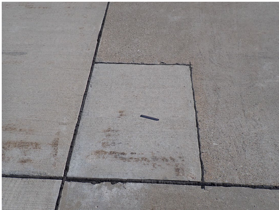
R16PE-10. Large Patching (Sample Unit No. 02).
