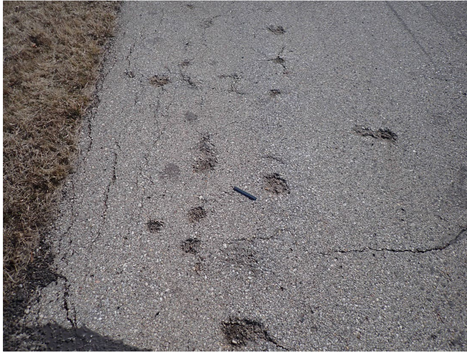
R171Y-02. Raveling (Sample Unit No. 04).
