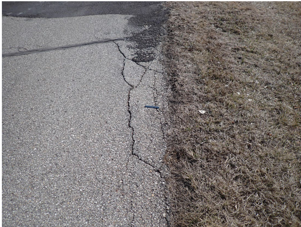
R171Y-02. Alligator Cracking (Sample Unit No. 06) (2).
