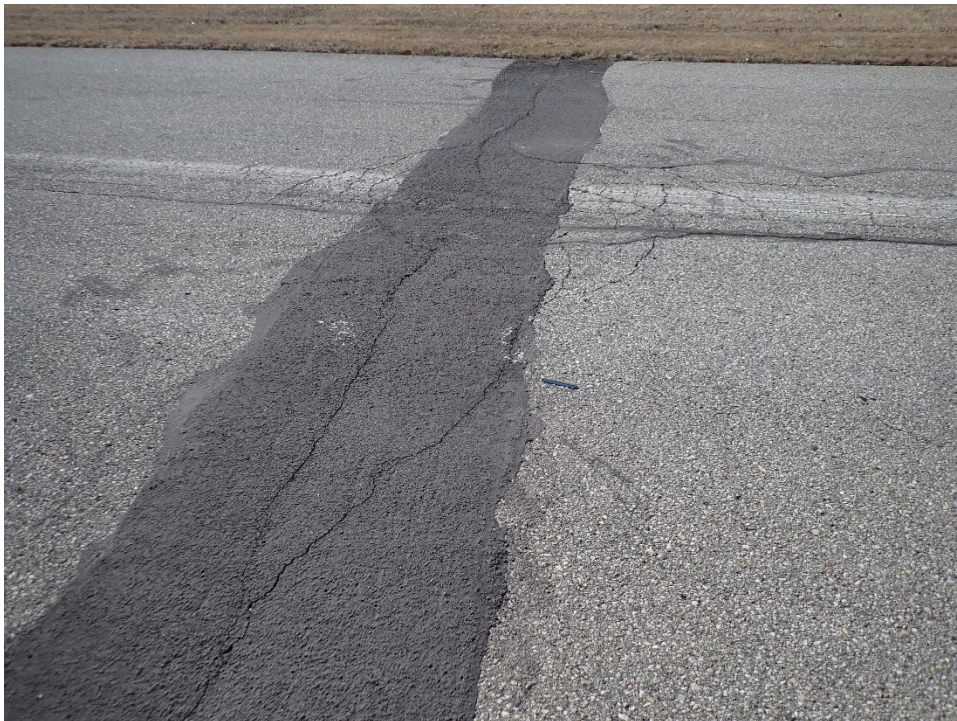
R171Y-02. Patching (Sample Unit No. 06).
