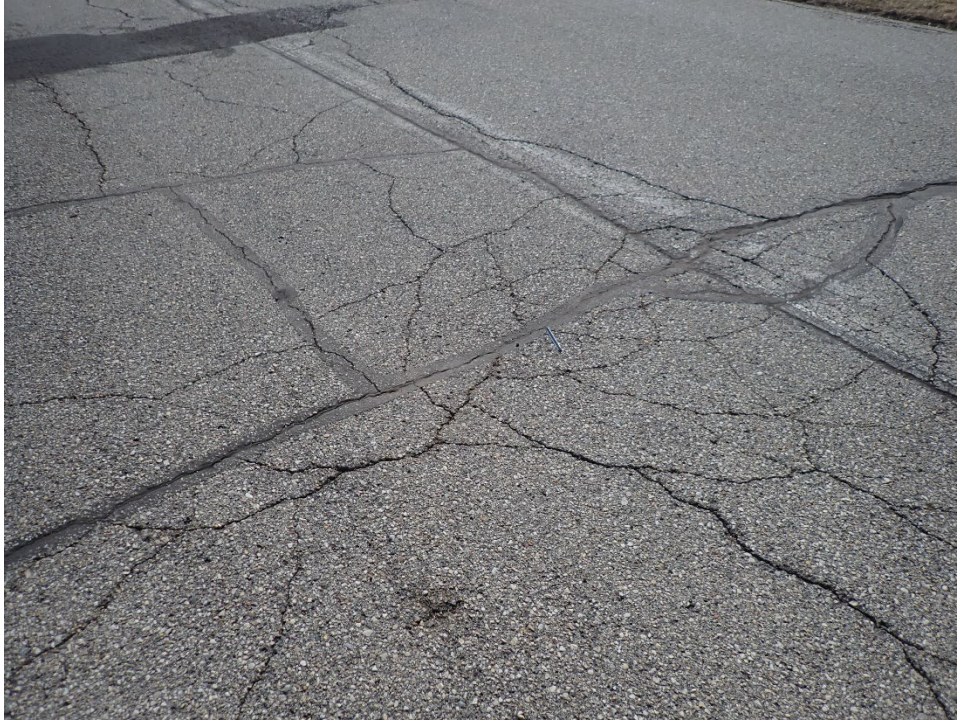
R171Y-03. Alligator Cracking (Sample Unit No. 01).
