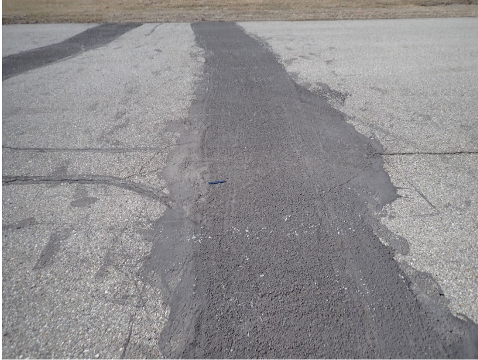
R171Y-01. Patching (Sample Unit No. 01).
