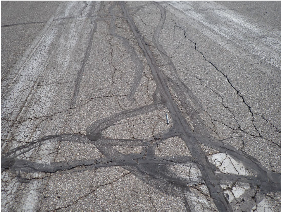
R171Y-01. Alligator Cracking (Sample Unit No. 01).
