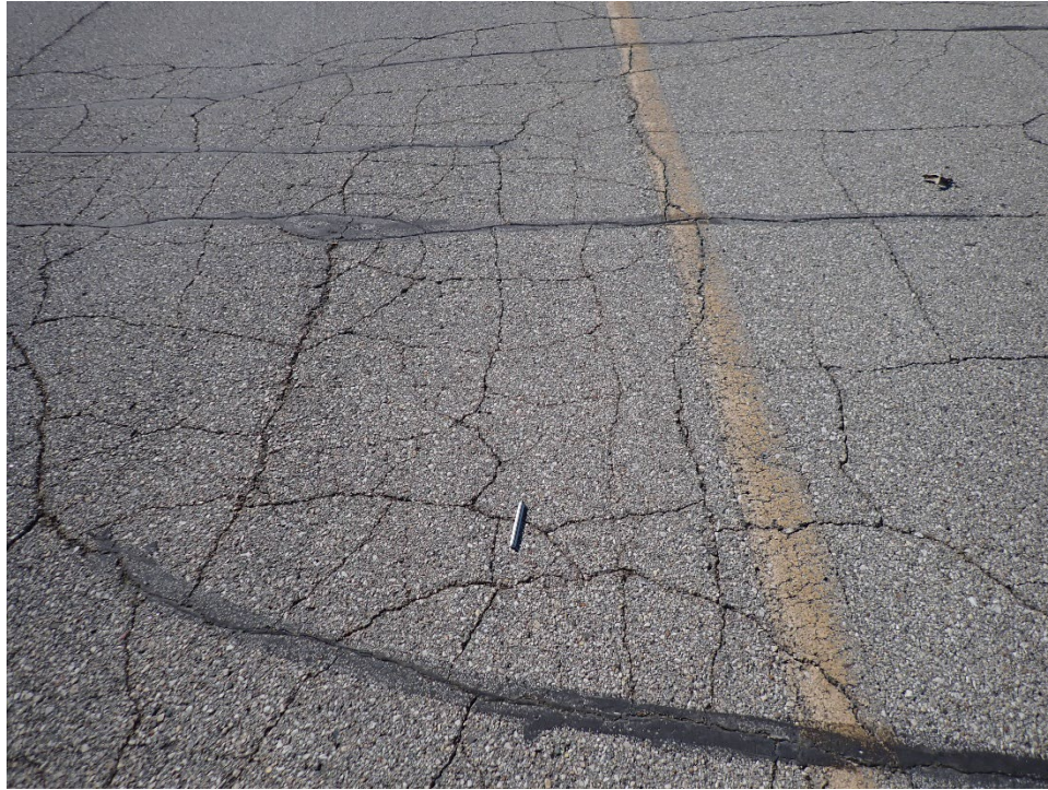
T011Y-01. Alligator Cracking (Sample Unit No. 01).
