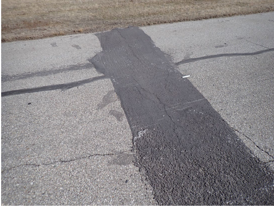
R171Y-02. Patching (Sample Unit No. 04).
