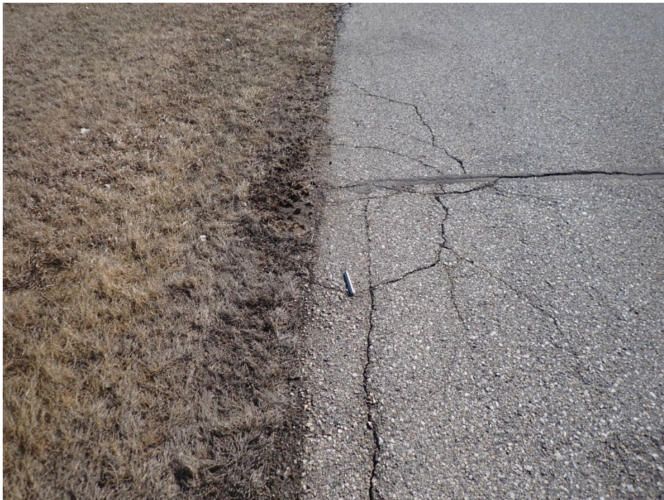
R171Y-03. Alligator Cracking (Sample Unit No. 02).
