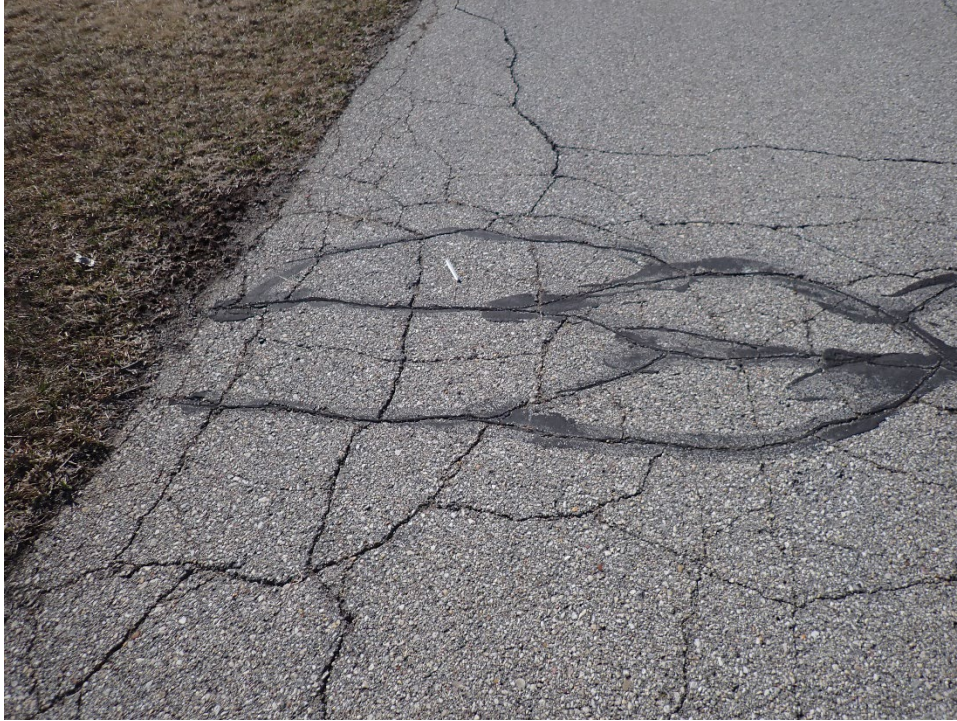
T011Y-03. Alligator Cracking (Sample Unit No. 01).
