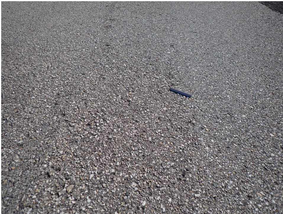
R171Y-03. Raveling (Sample Unit No. 03) (1).
