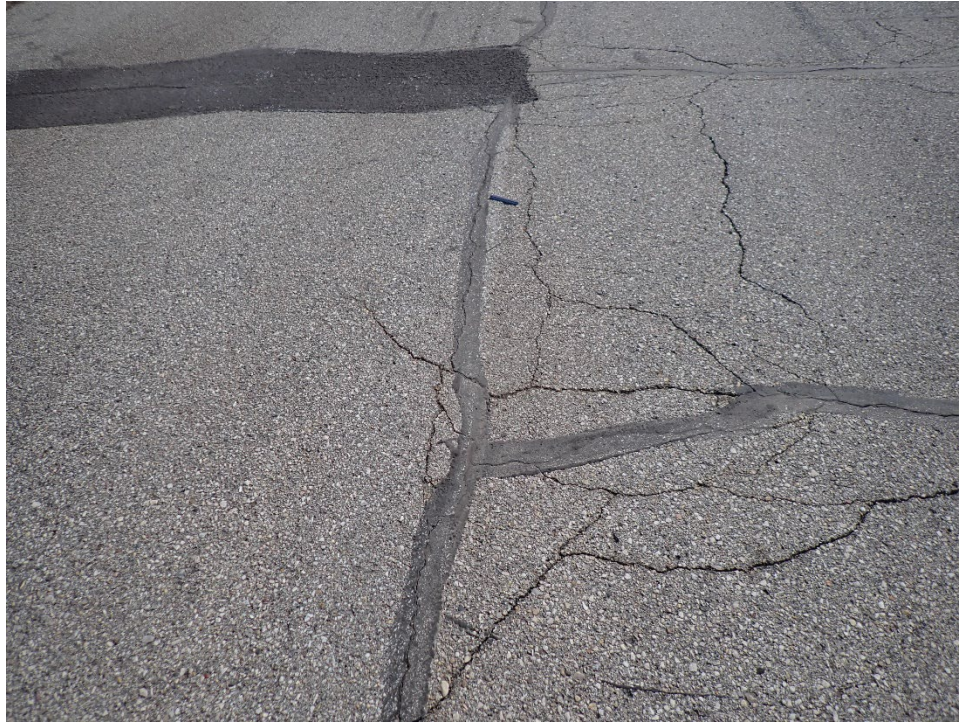
R171Y-02. Alligator Cracking (Sample Unit No. 06) (1).
