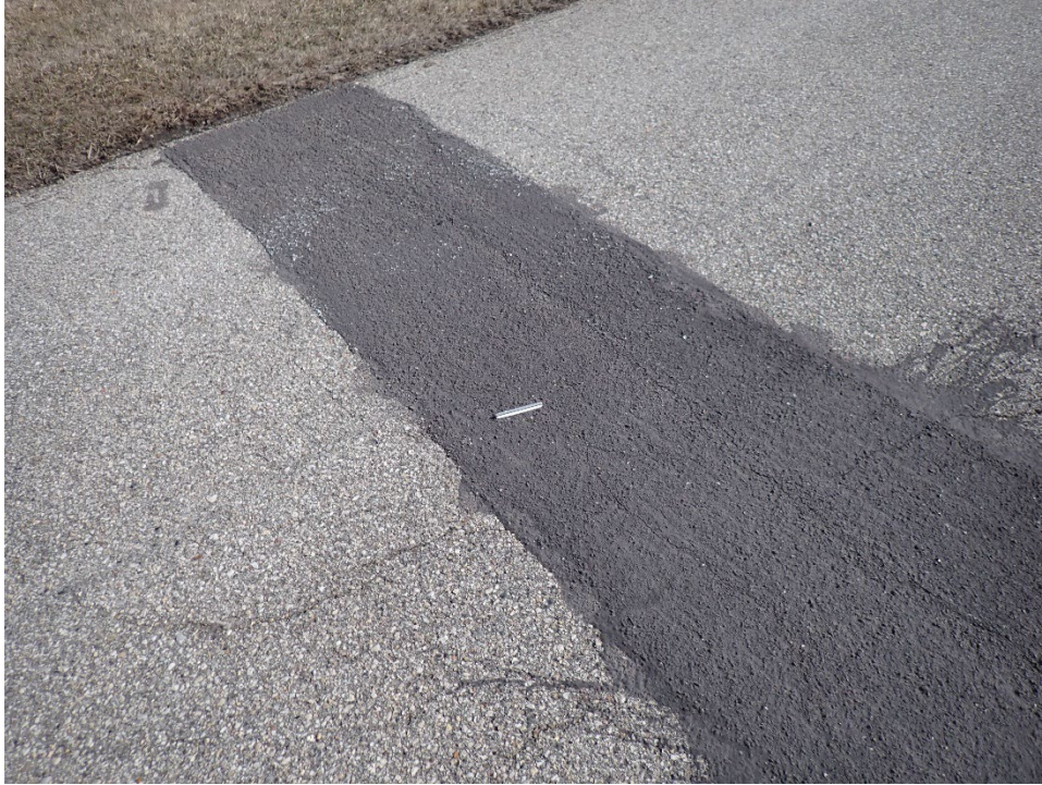
R171Y-03. Patching (Sample Unit No. 02).
