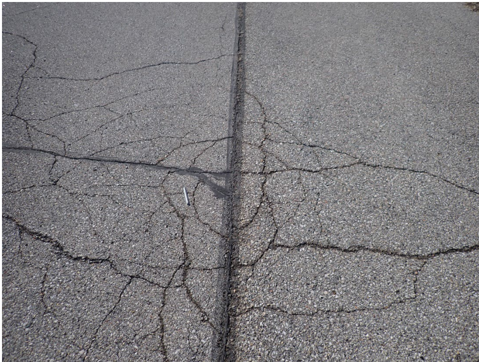
T011Y-02. Alligator Cracking (Sample Unit No. 01).
