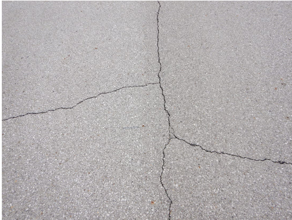
TAOT-02. L&T Cracking (Sample Unit No. 01).
