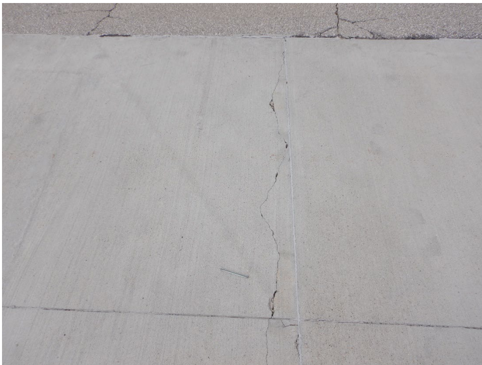
A01OT-09. Joint Spalling (Sample Unit No. 02).
