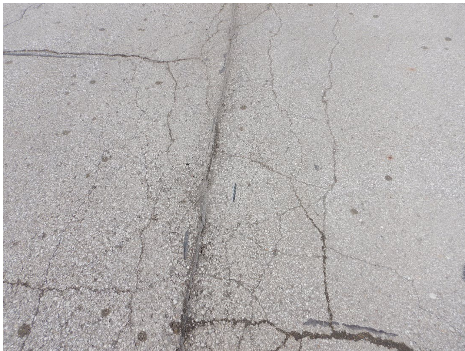
A02OT-03. Alligator Cracking (Sample Unit No. 01).
