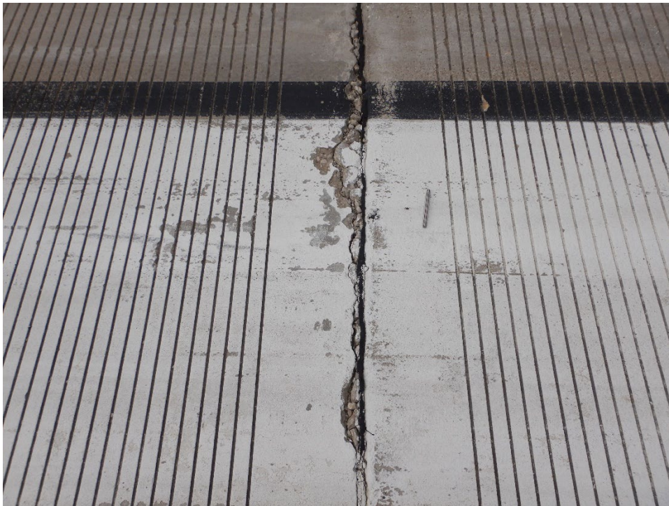
R13OT-01. Joint Spalling (Sample Unit No. 06).
