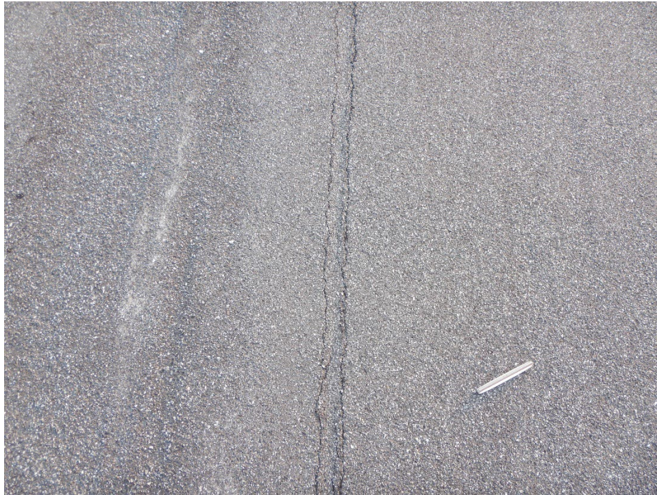
R04OT-03. L&T Cracking (Sample Unit No. 08).
