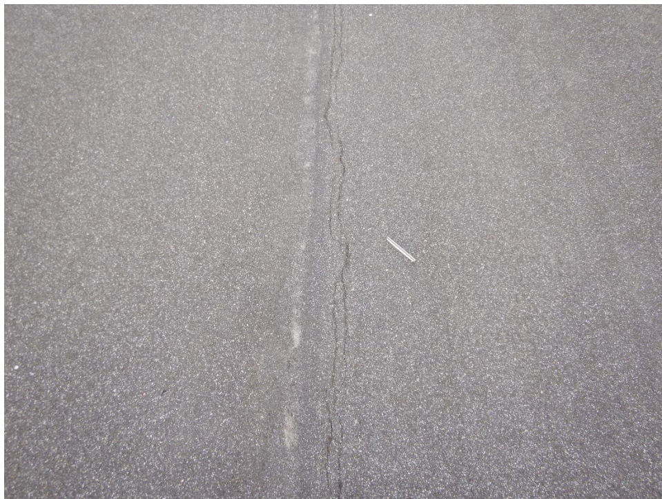
TBOT-04. L&T Cracking (Sample Unit No. 02) (2).
