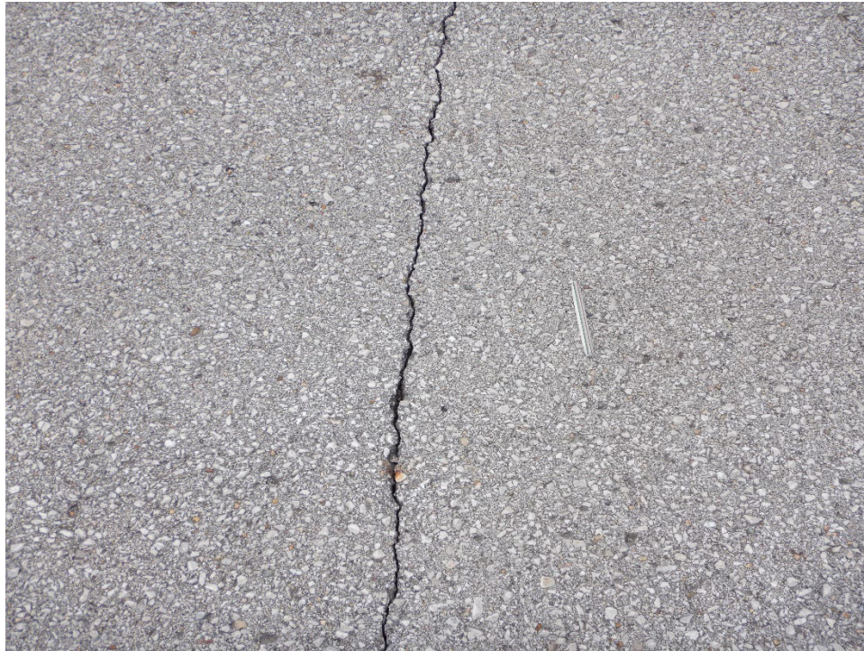
TAOT-04. L&T Cracking (Sample Unit No. 01) (2).
