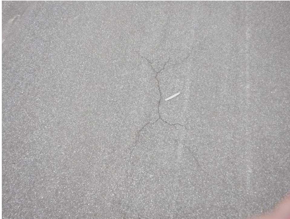
TBOT-04. L&T Cracking (Sample Unit No. 02) (1).
