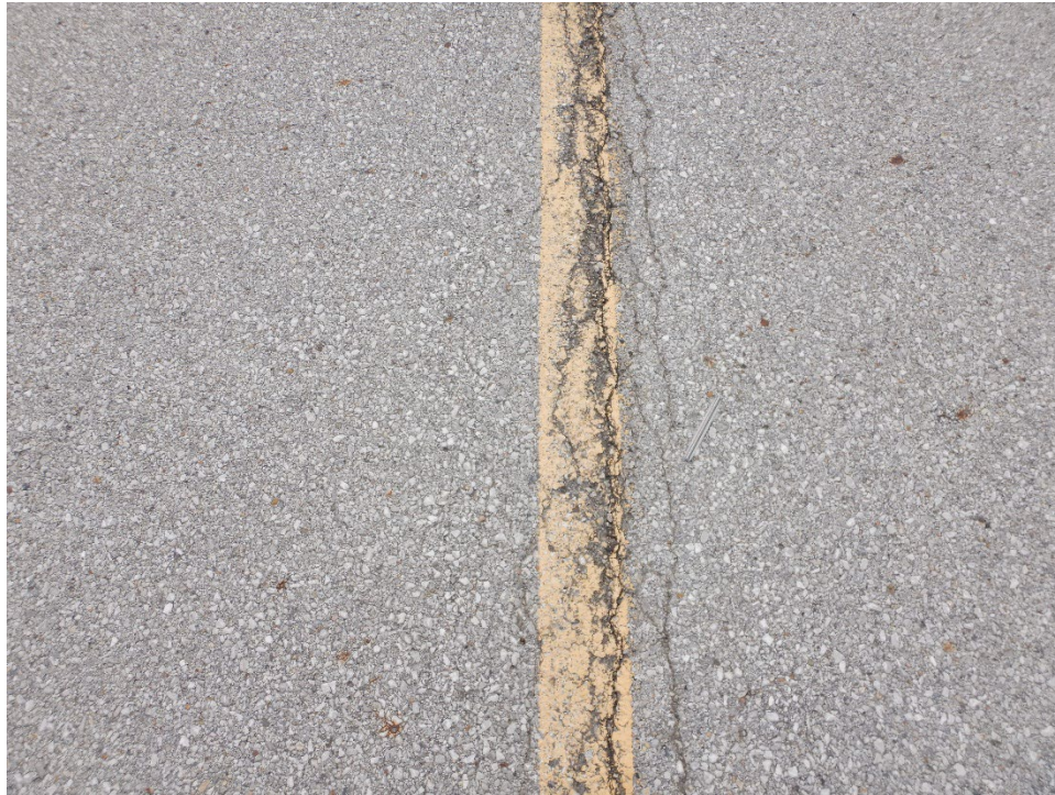
TAOT-01. L&T Cracking (Sample Unit No. 11).
