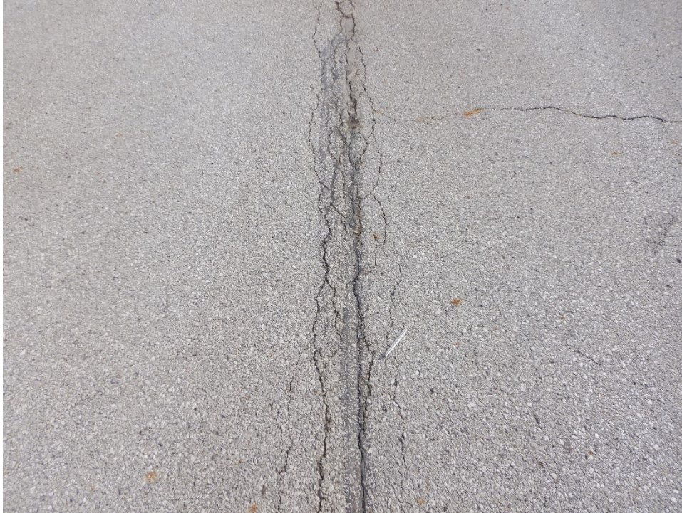
A02OT-02. L&T Cracking (Sample Unit No. 10).
