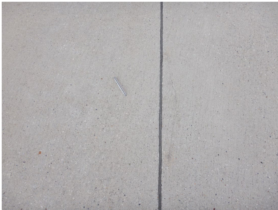
TAOT-08. Joint Spalling (Sample Unit No. 18).
