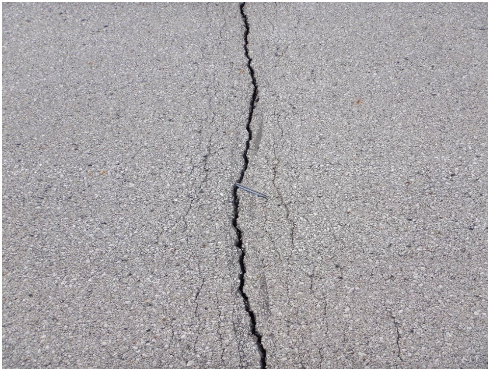
A02OT-02. L&T Cracking (Sample Unit No. 14).
