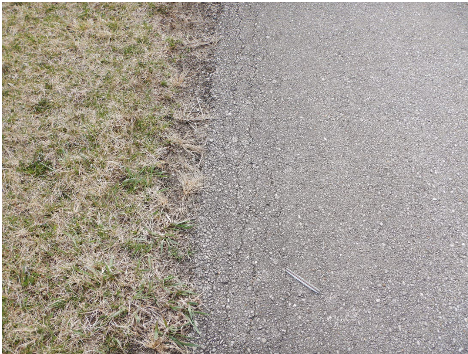
TAOT-03. Alligator Cracking (Sample Unit No. 03).
