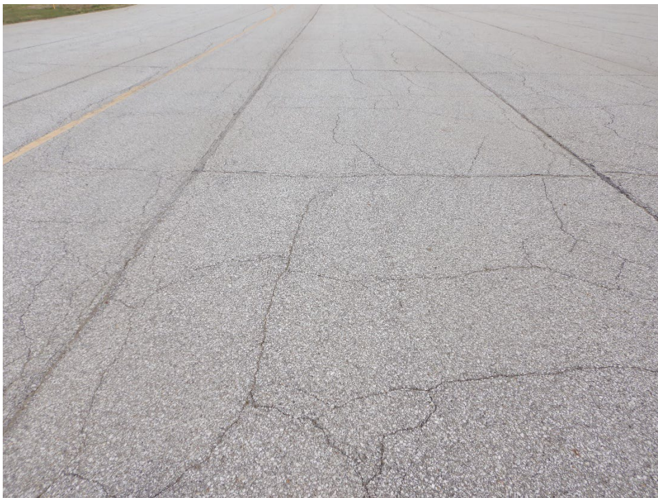
A01OT-02. Block Cracking (Sample Unit No. 02).
