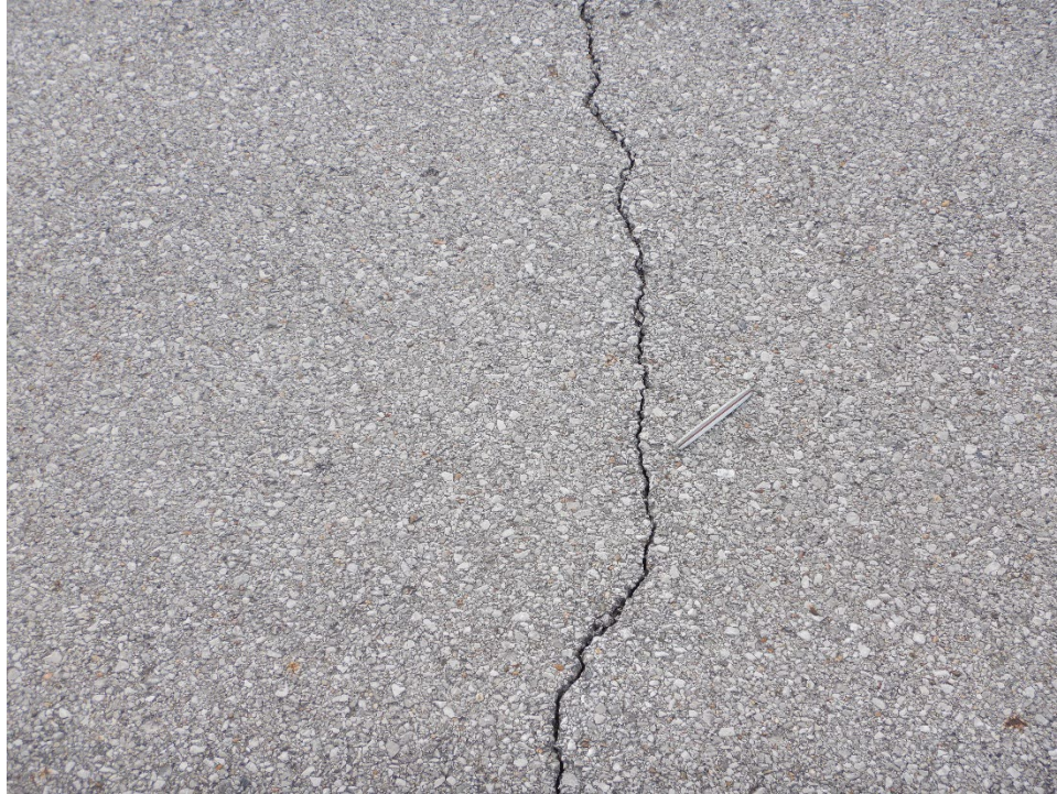
TBOT-02. L&T Cracking (Sample Unit No. 01).
