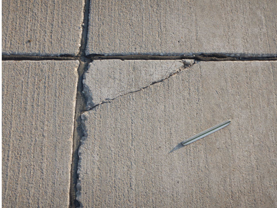
R04OT-04. Corner Spalling (Sample Unit No. 04).
