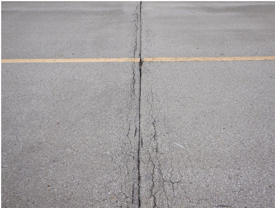
TAOT-04. L&T Cracking (Sample Unit No. 01) (1).
