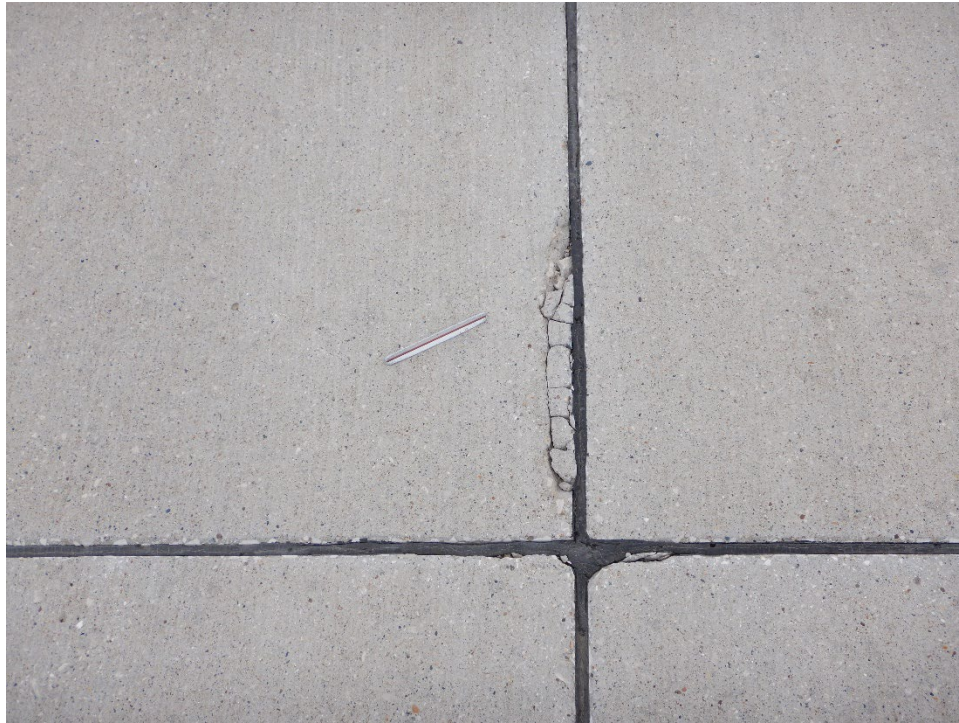
TAOT-08. Joint Spalling (Sample Unit No. 12).
