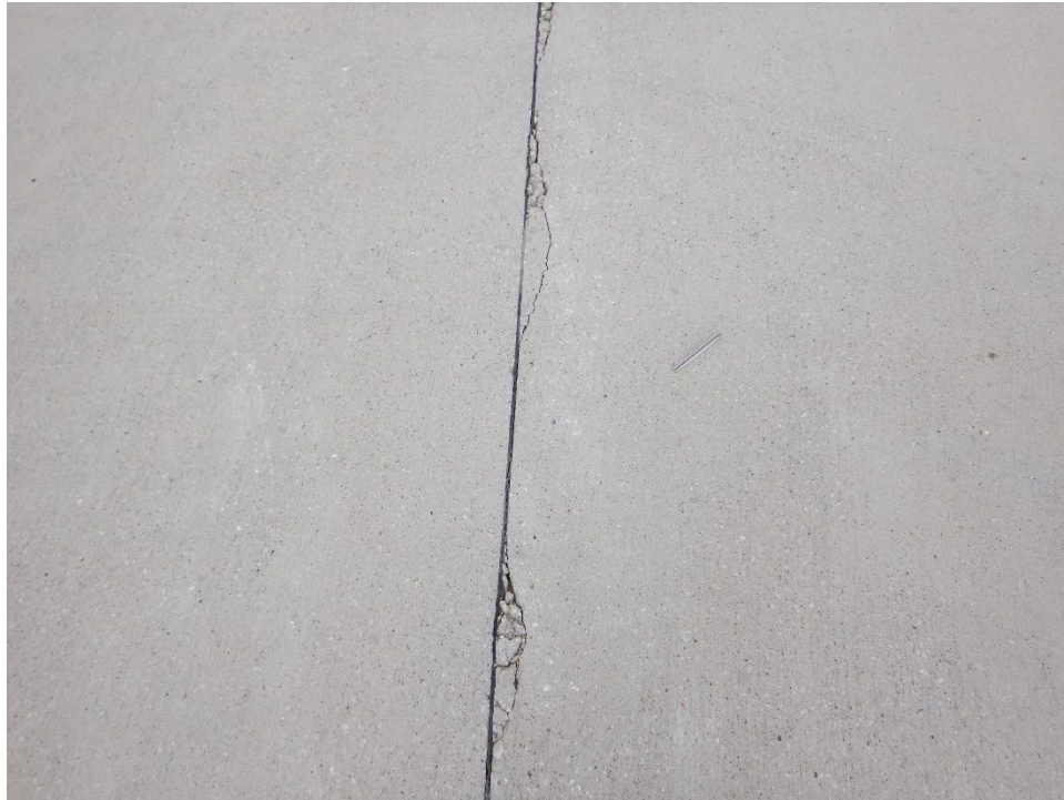
A01OT-07. Joint Spalling (Sample Unit No. 15).
