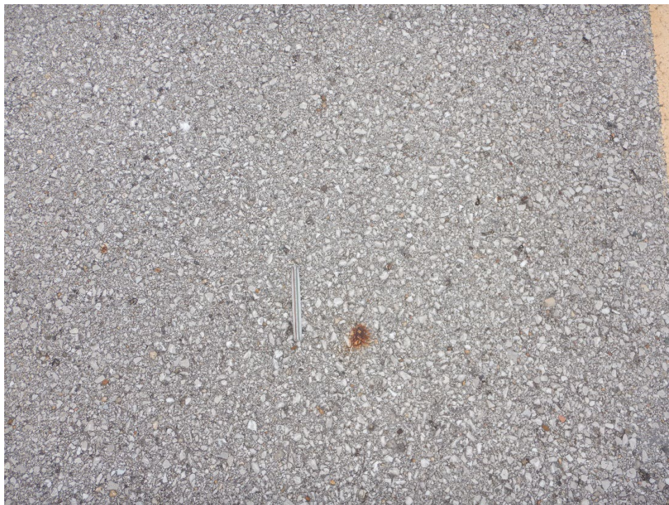
TAOT-04. Raveling (Sample Unit No. 01).
