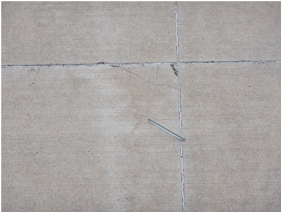
A01OT-06. Corner Spalling (Sample Unit No. 14).
