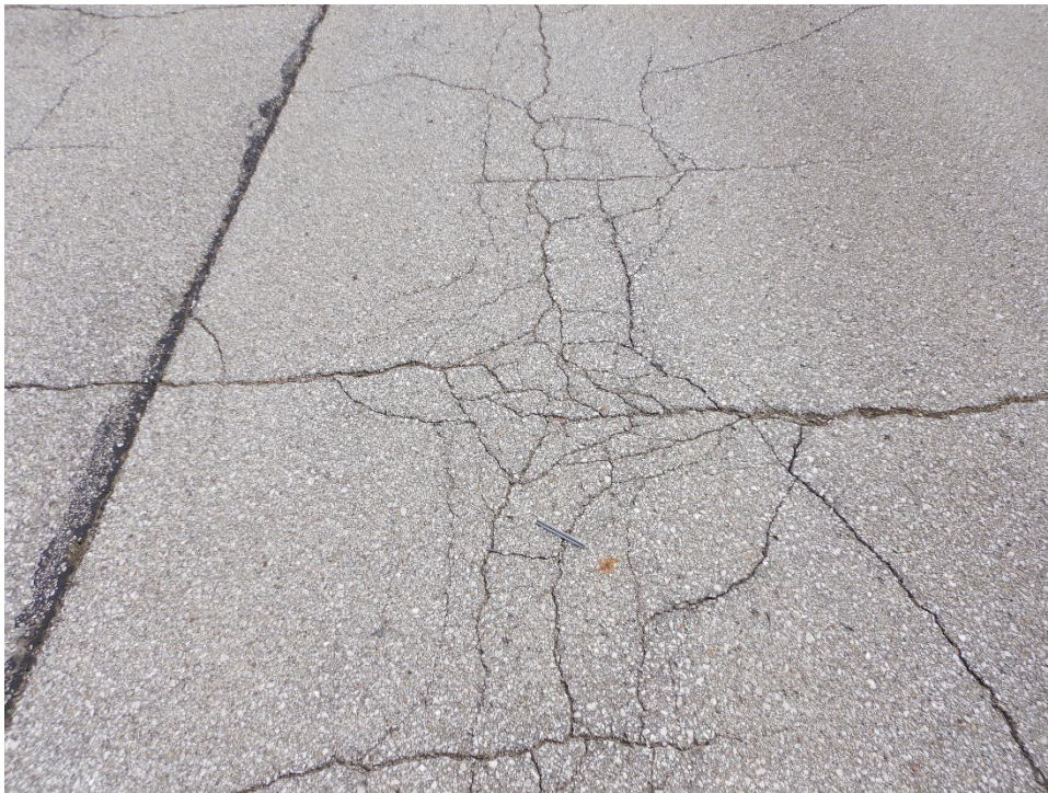
TAOT-06. Alligator Cracking (Sample Unit No. 06).
