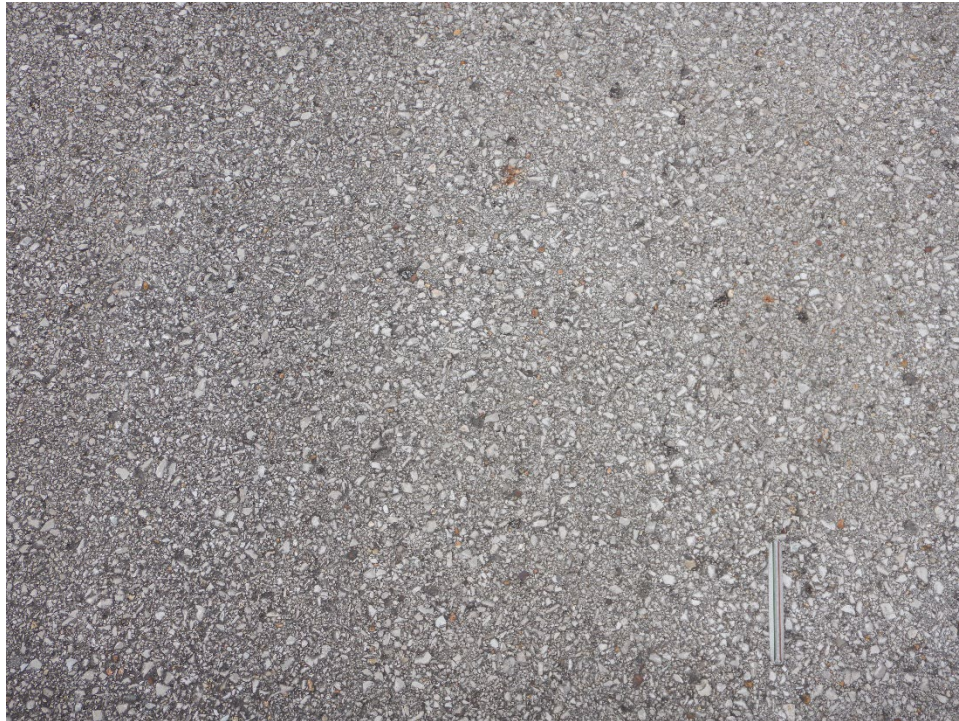
TAOT-05. Raveling (Sample Unit No. 01) (2).
