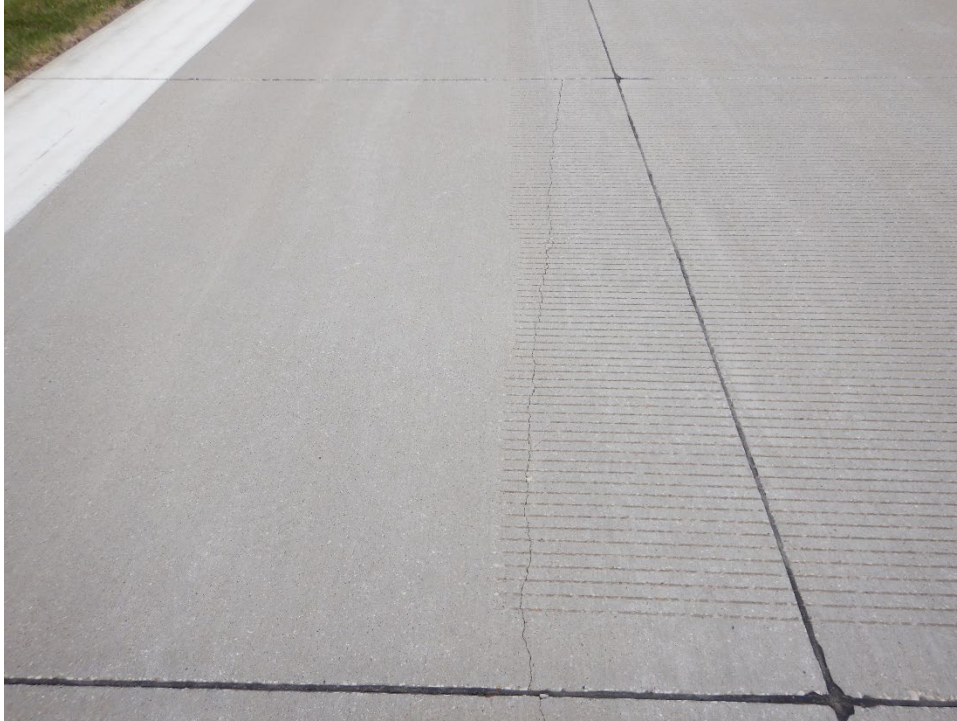
R13OT-01. LTD Cracking (Sample Unit No. 186).
