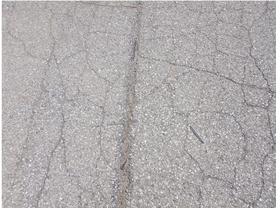
A01OT-04. Alligator Cracking (Sample Unit No. 02).
