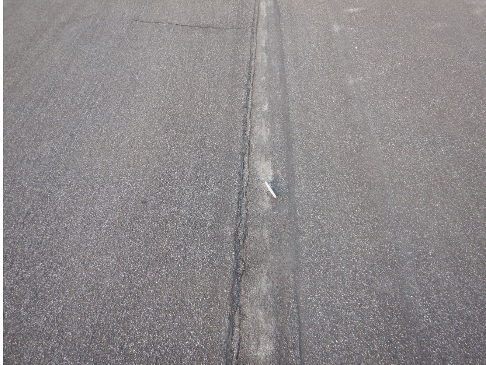
R04OT-02. Joint Reflection Cracking (Sample Unit No. 65).
