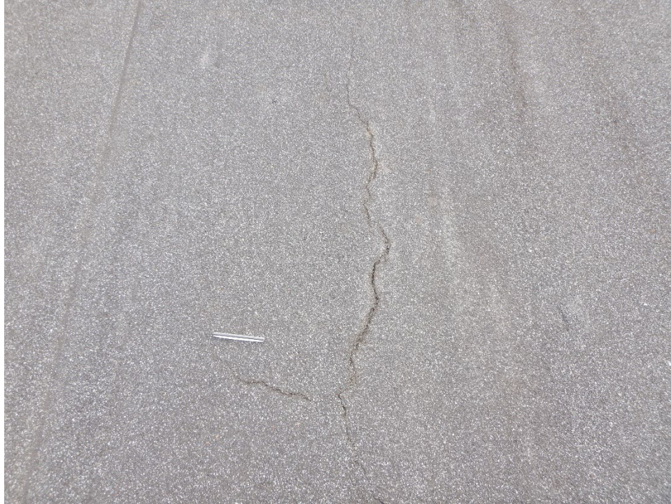
TBOT-03. L&T Cracking (Sample Unit No. 06).
