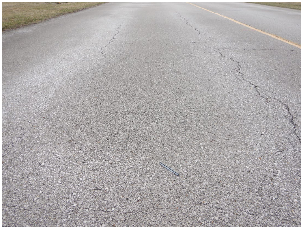
TAOT-03. Rutting (Sample Unit No. 09).
