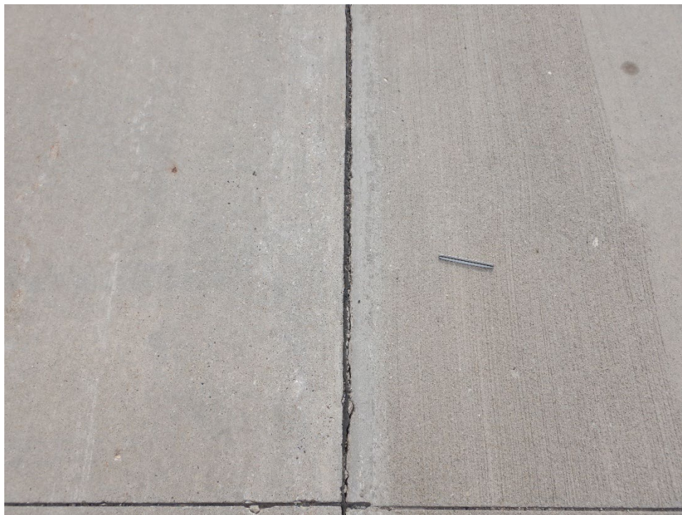
A01OT-07. Joint Seal Damage (Sample Unit No. 11).
