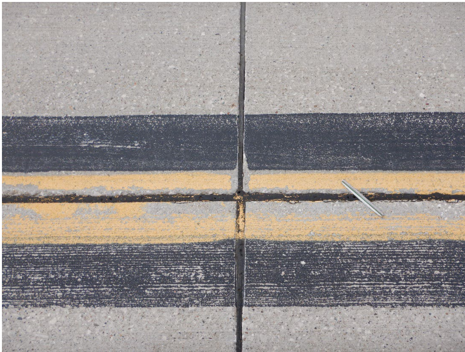
TAOT-08. Joint Seal Damage (Sample Unit No. 21).
