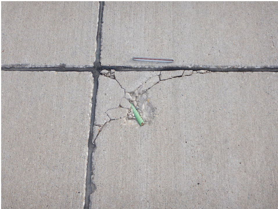
TBOT-07. Corner Spalling (Sample Unit No. 02).
