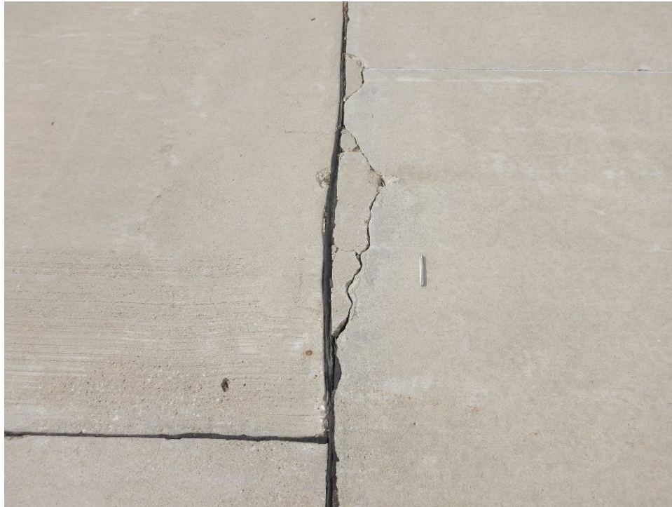
A01OT-08. Joint Spalling (Additional Sample Unit No. 11).
