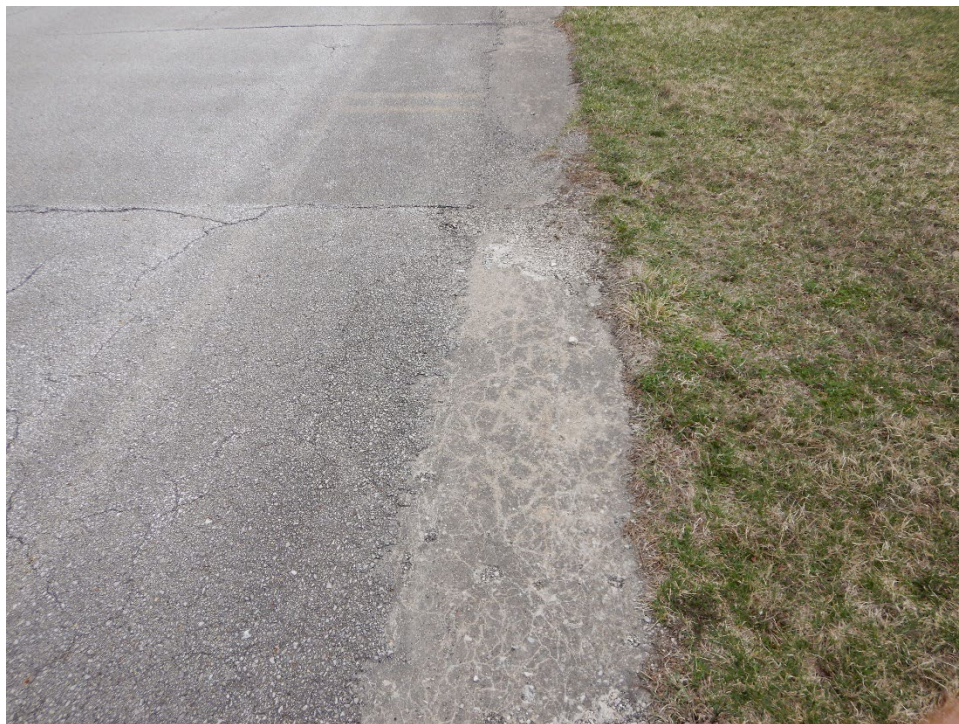
TAOT-02. Patching (Sample Unit No. 01).
