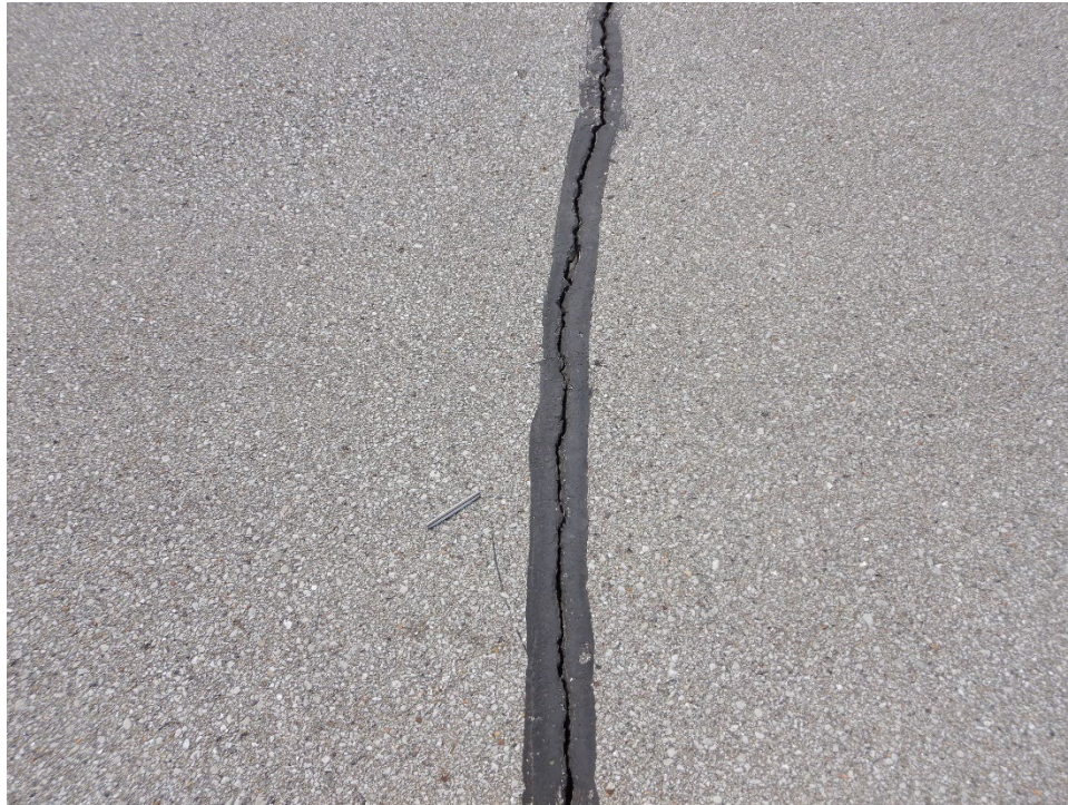
A02OT-03. L&T Cracking (Sample Unit No. 01).
