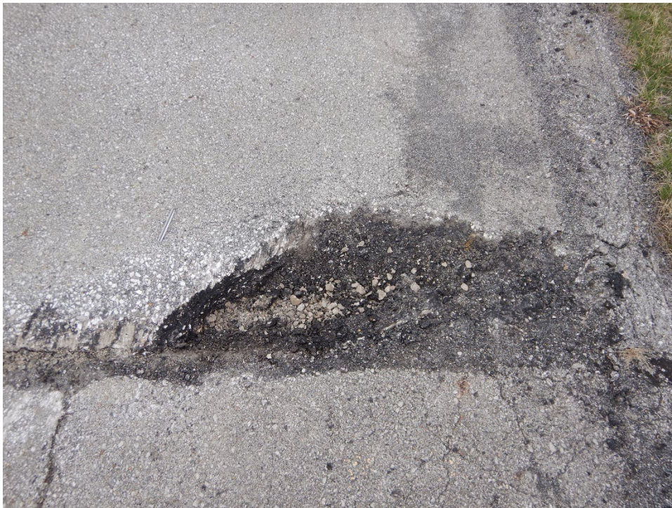
TAOT-05. Raveling (Sample Unit No. 01) (1).
