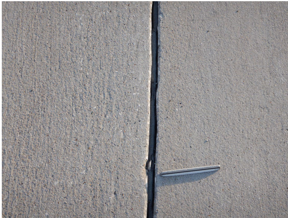
R04OT-04. Joint Seal Damage (Sample Unit No. 01).
