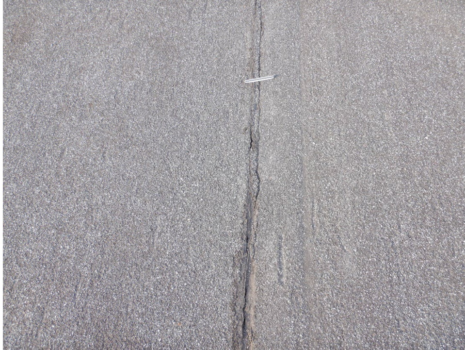
R04OT-01. Joint Reflection Cracking (Sample Unit No. 06).
