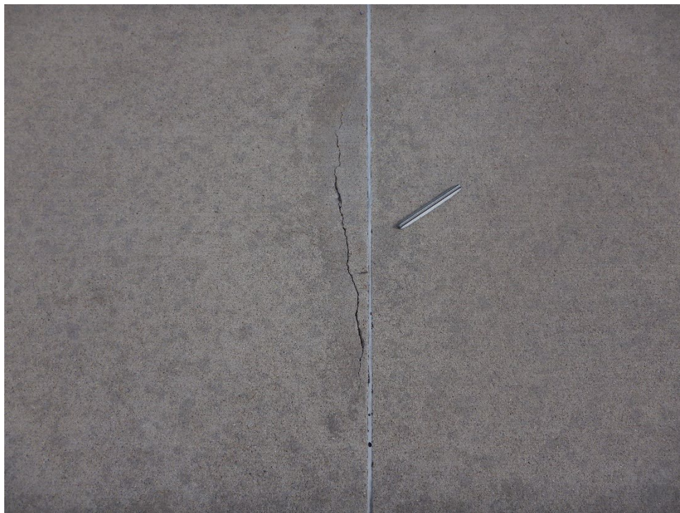
A01OT-08. Joint Spalling (Sample Unit No. 04).
