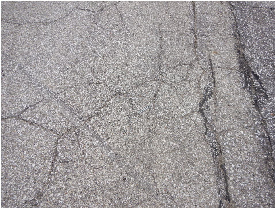
TBOT-01. Alligator Cracking (Sample Unit No. 02).
