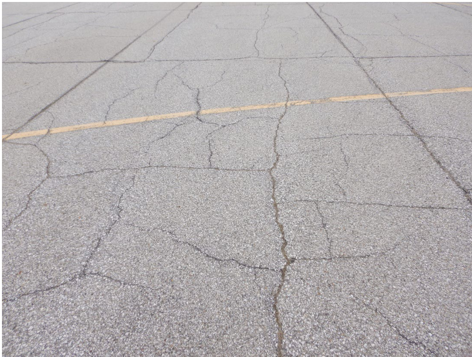
A02OT-01. Block Cracking (Sample Unit No. 02).
