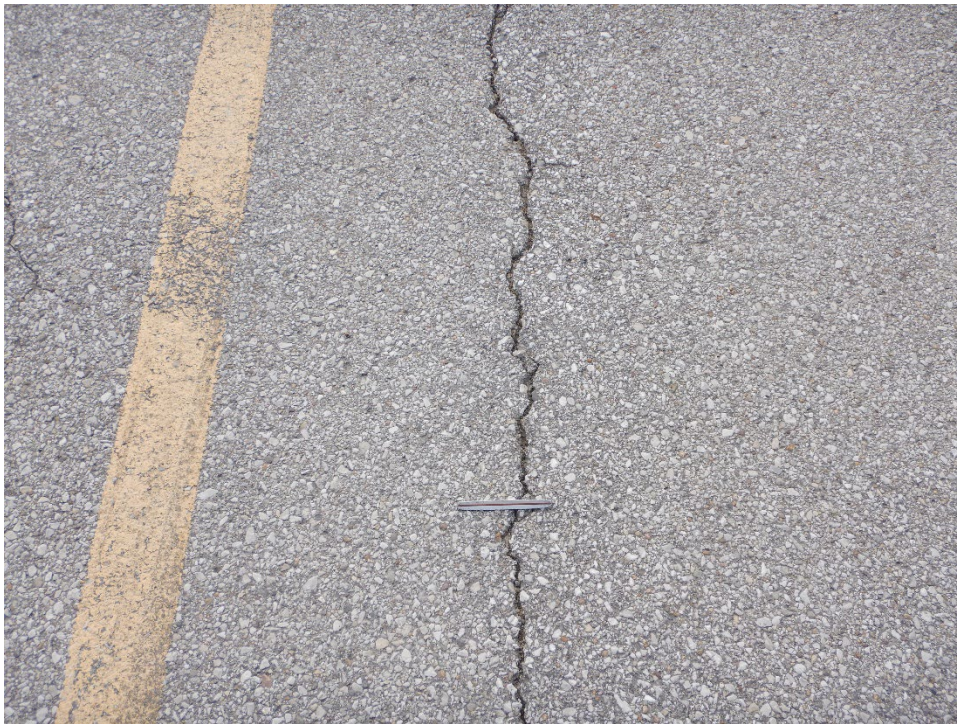
TBOT-06. L&T Cracking (Sample Unit No. 01).
