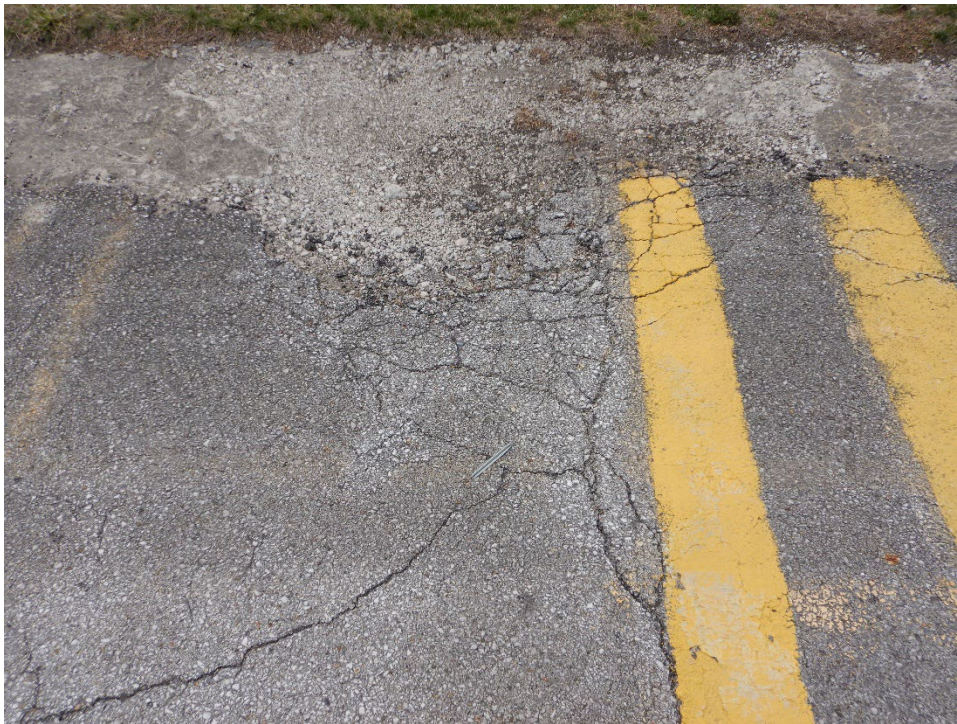
TAOT-02. Alligator Cracking (Sample Unit No. 01).
