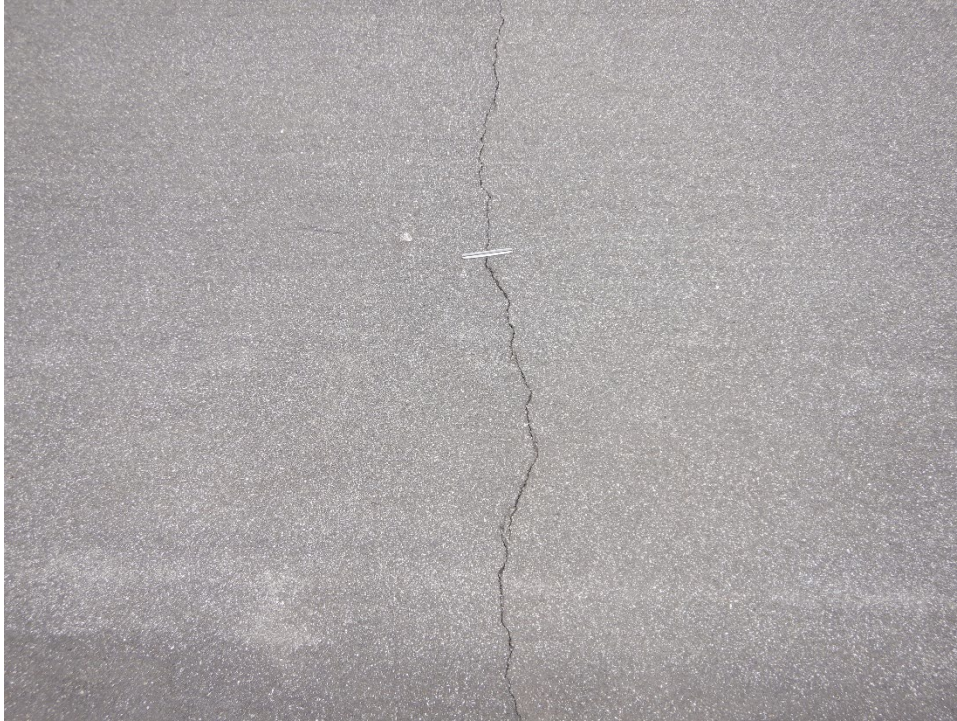
TCOT-01. L&T Cracking (Sample Unit No. 02).
