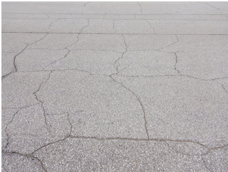
A01OT-01. Block Cracking (Sample Unit No. 04).
