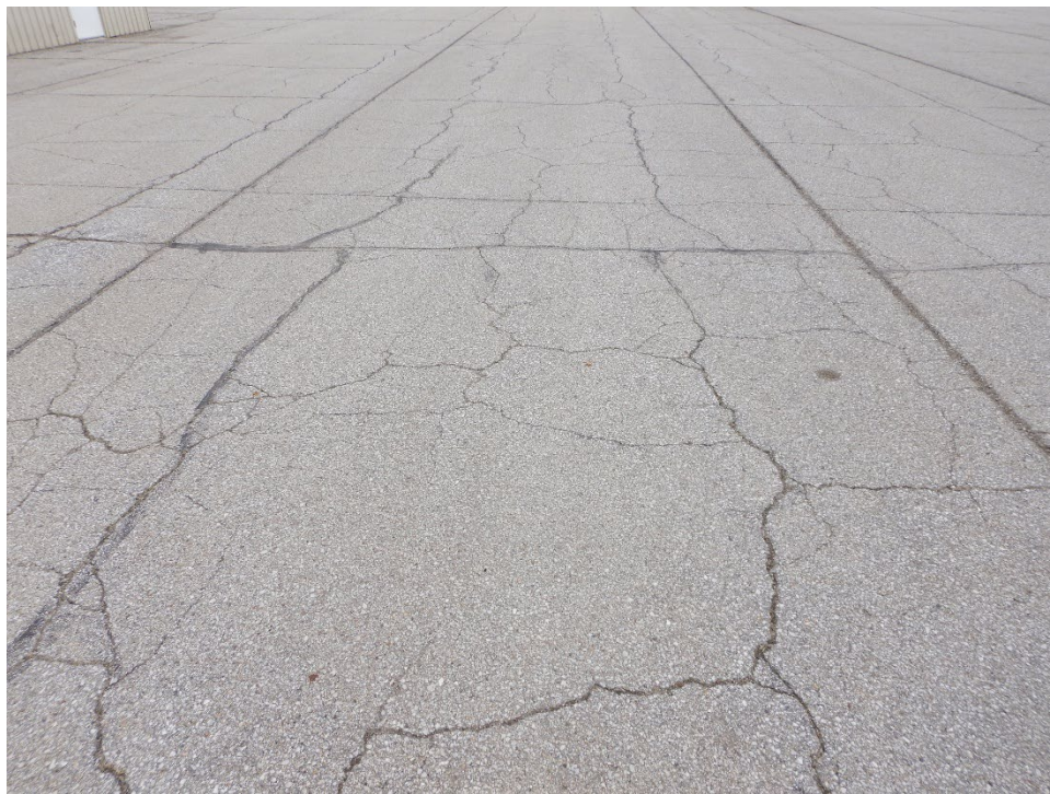
A01OT-05. Block Cracking (Sample Unit No. 02).
