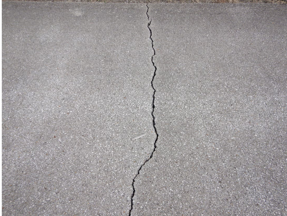
TAOT-03. L&T Cracking (Sample Unit No. 03).
