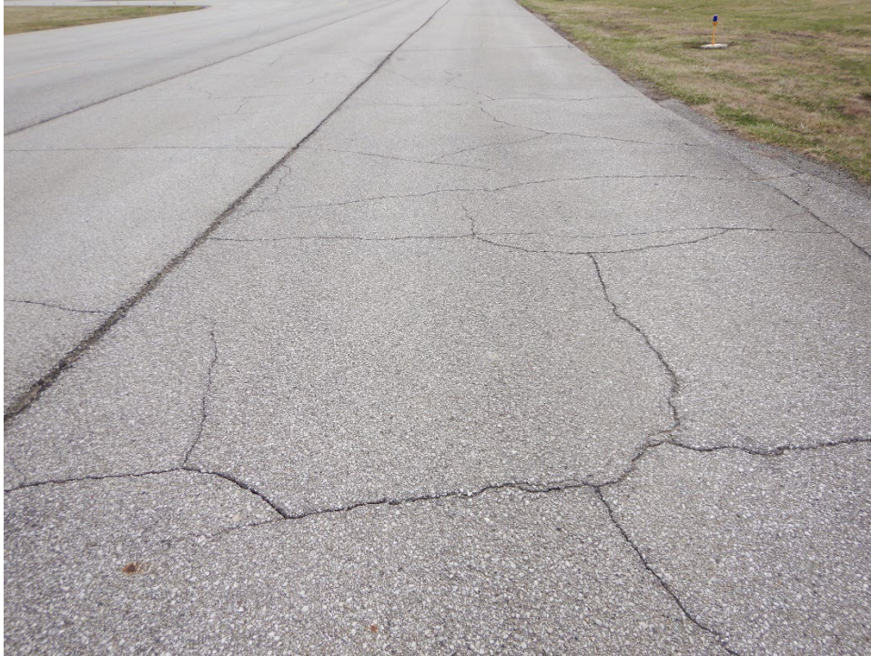
TBOT-01. Block Cracking (Sample Unit No. 03).
