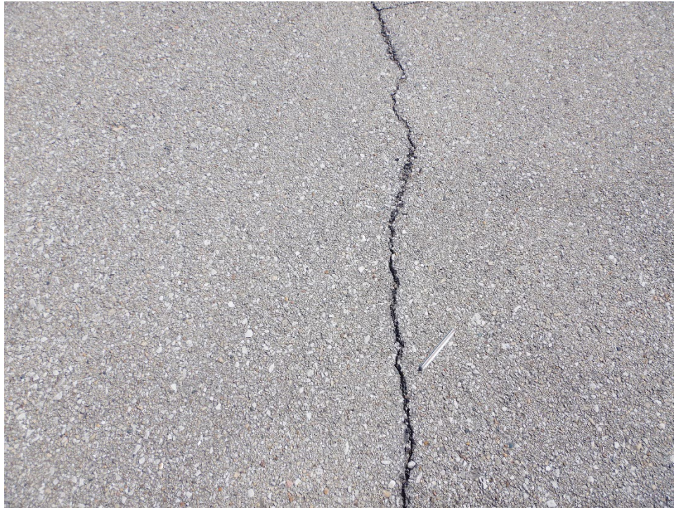
A02OT-04. L&T Cracking (Sample Unit No. 01).
