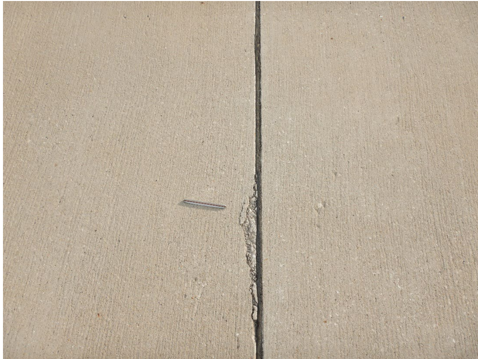
TBOT-07. Joint Spalling (Sample Unit No. 10).
