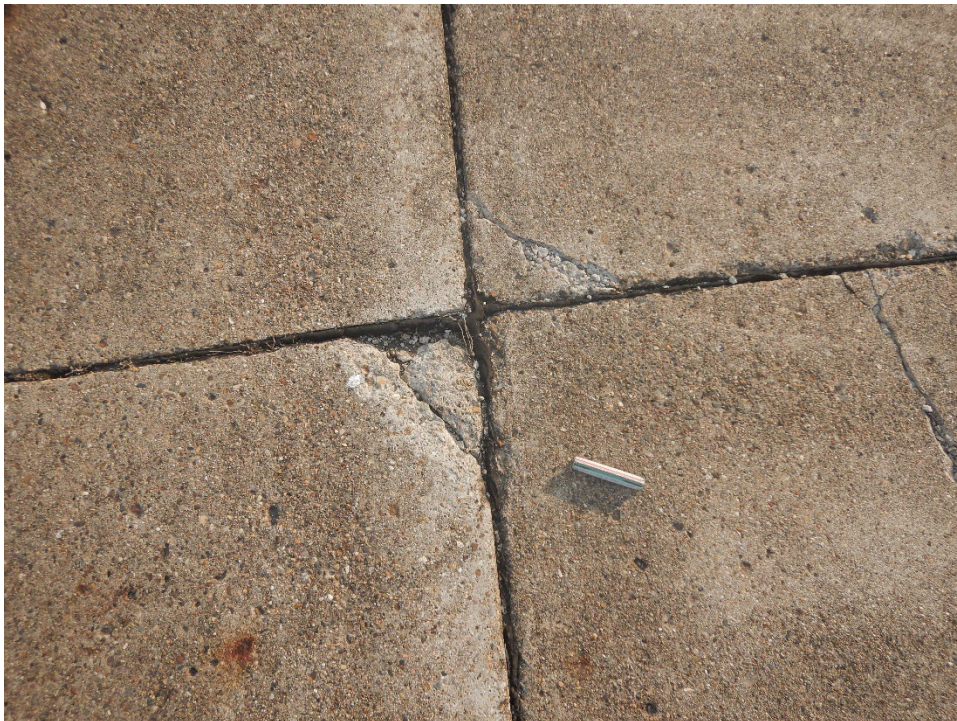
T01OK-01. Corner Spalling (Sample Unit No. 08).
