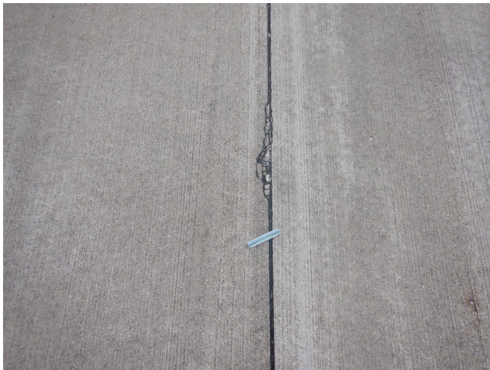
T02OK-01. Joint Spalling (Sample Unit No. 05).
