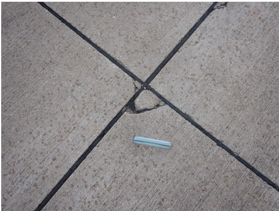
T03OK-01. Corner Spalling (Sample Unit No. 02).
