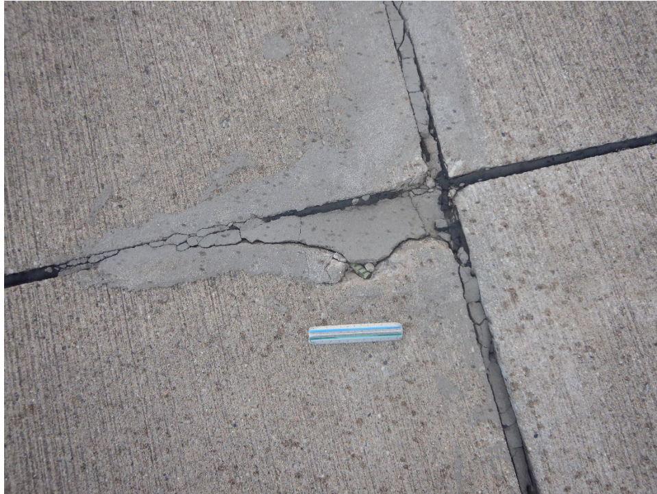
T03OK-01. Small Patching (Sample Unit No. 02).
