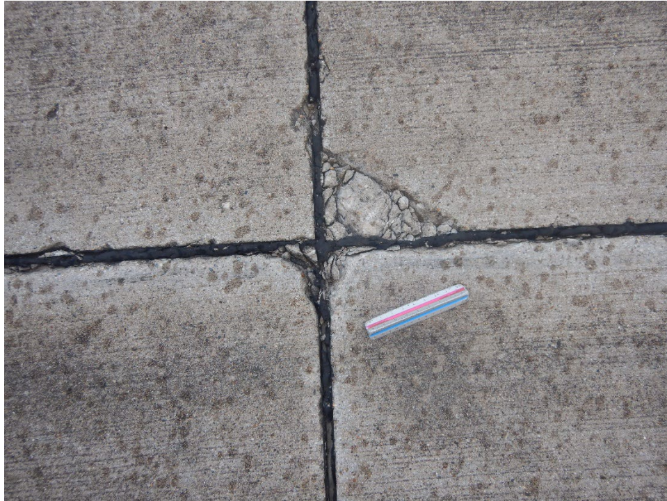
T04OK-01. Corner Spalling (Sample Unit No. 03).
