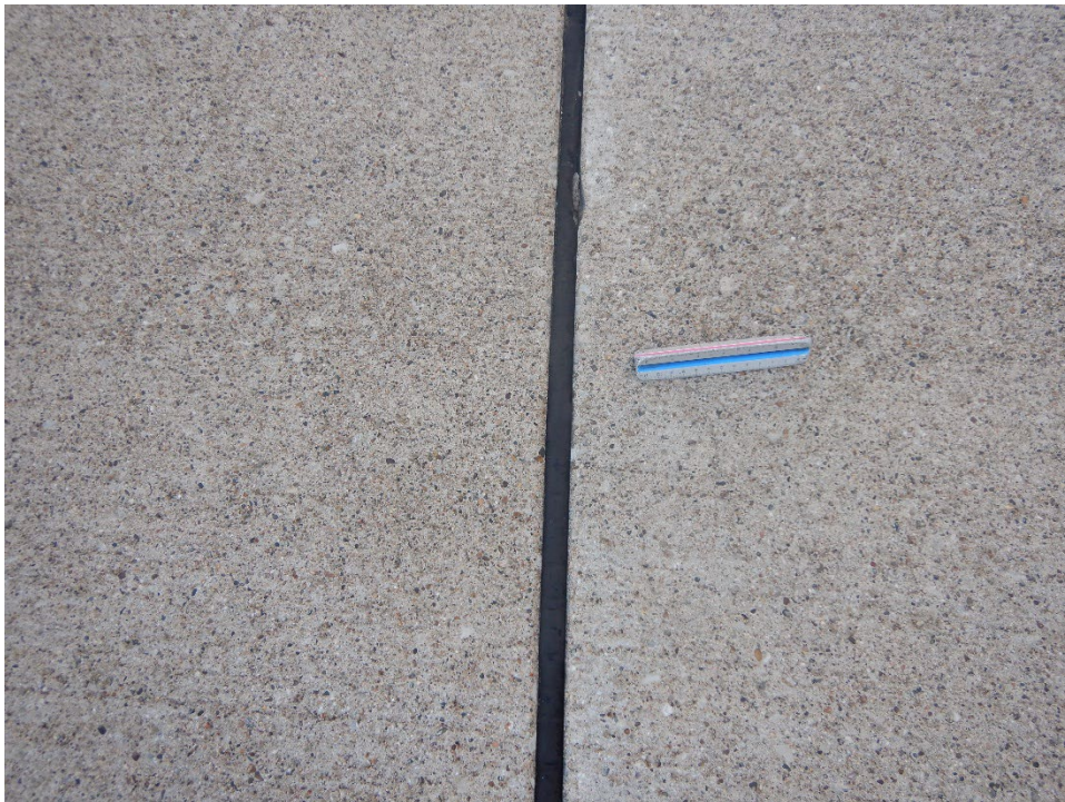
T05OK-02. Joint Seal Damage (Sample Unit No. 19).
