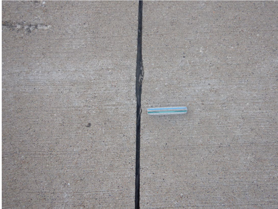
T02OK-01. Joint Seal Damage (Sample Unit No. 05).
