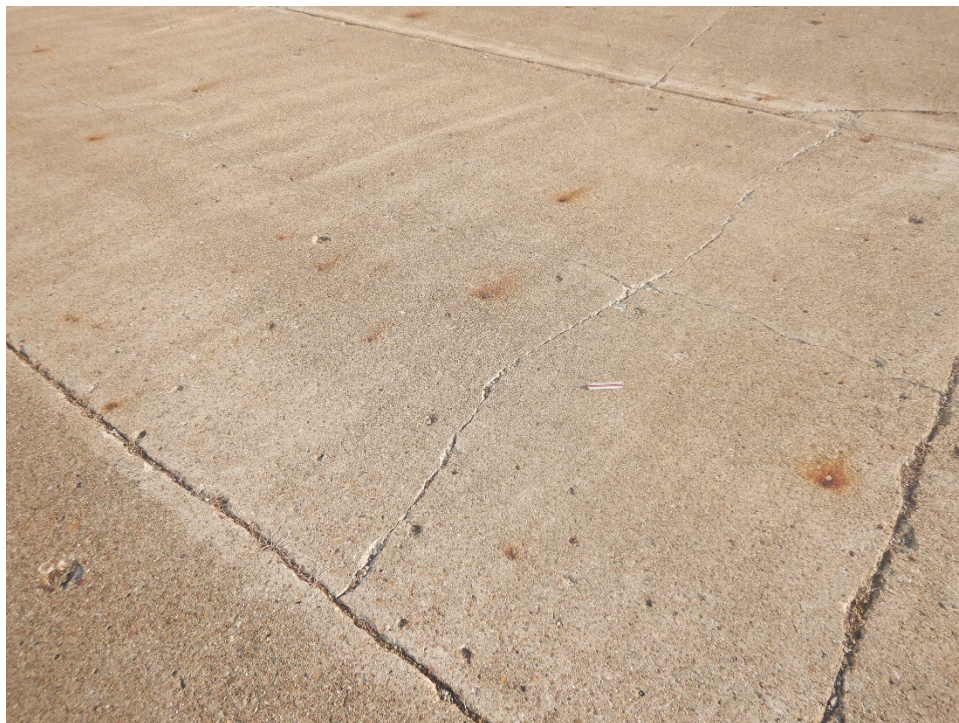
TH01OK-01. Shattered Slab (Sample Unit No. 02).
