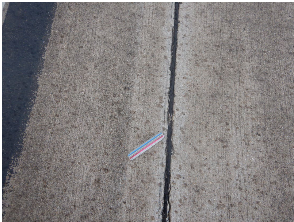
T04OK-01. Joint Seal Damage (Sample Unit No. 03).
