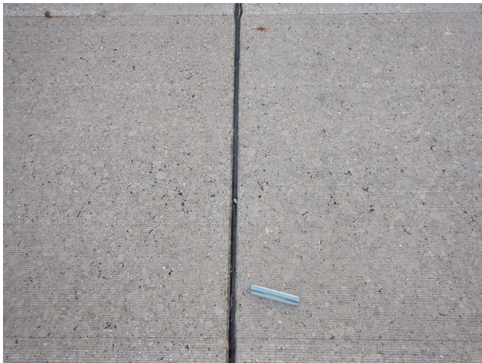
T05OK-03. Joint Seal Damage (Sample Unit No. 12).
