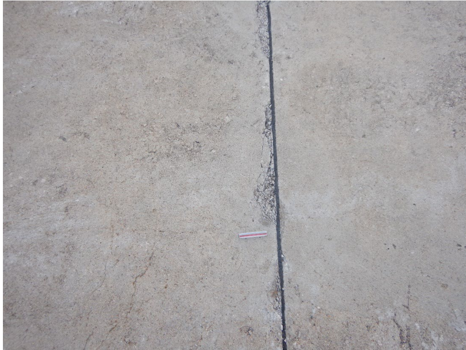
T05OK-03. Joint Spalling (Sample Unit No. 01).
