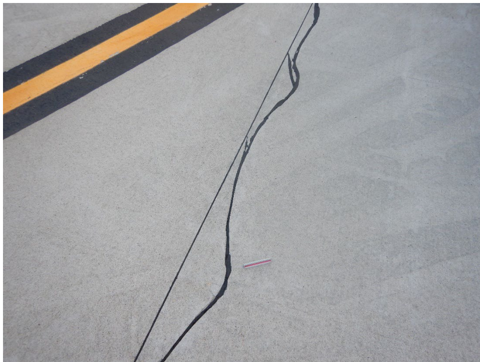
T01OK-02. Joint Spalling (Sample Unit No. 01).
