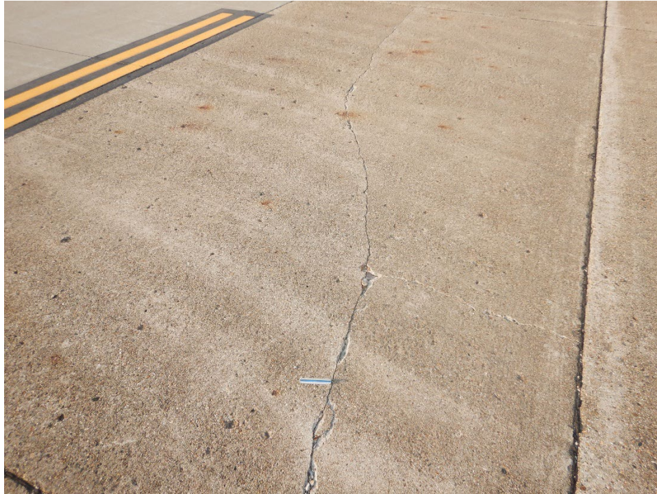
T01OK-01. LTD Cracking (Sample Unit No. 08).
