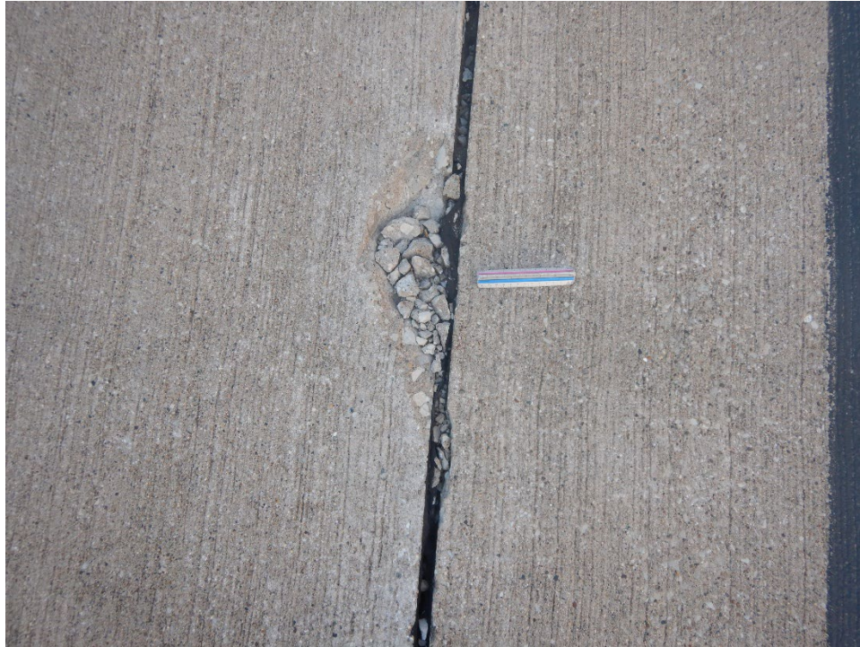
R13OK-01. Joint Spalling (Sample Unit No. 01).
