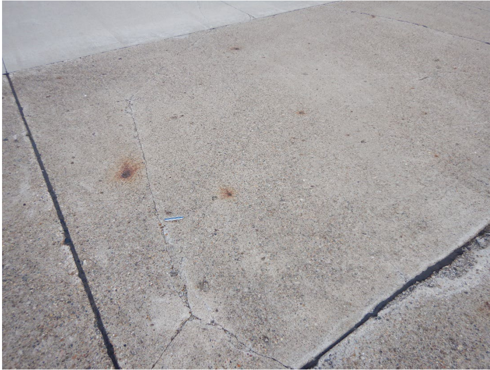
R04OK-01. Shattered Slab (Sample Unit No. 04).
