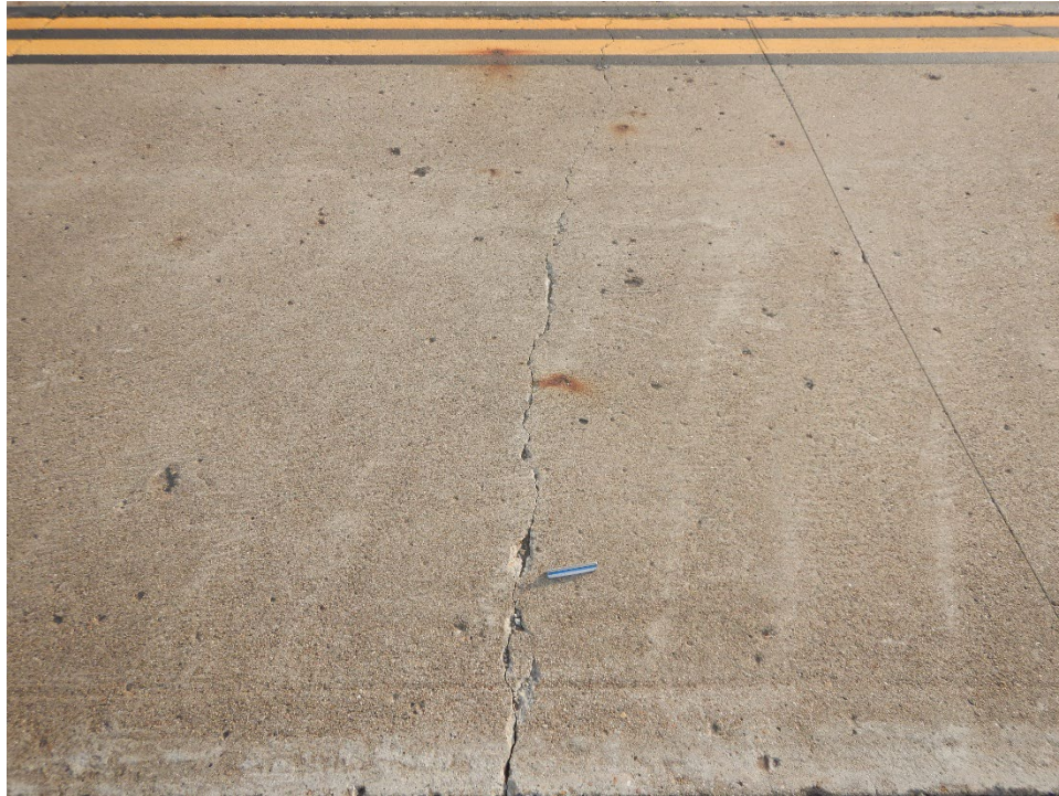
T01OK-03. LTD Cracking (Sample Unit No. 02).
