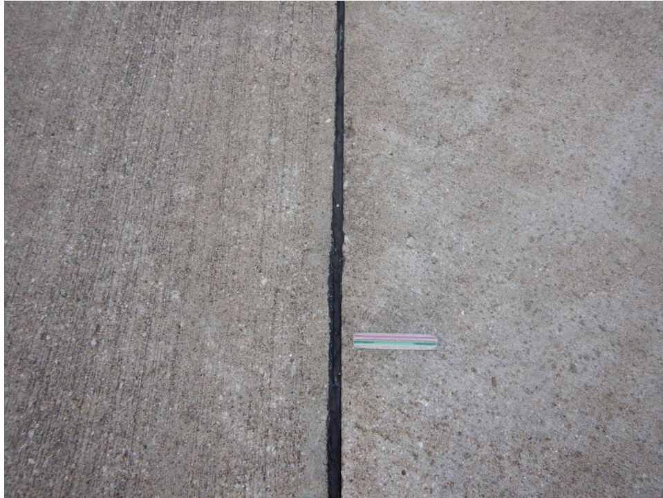
T01OK-02. Joint Seal Damage (Sample Unit No. 01).
