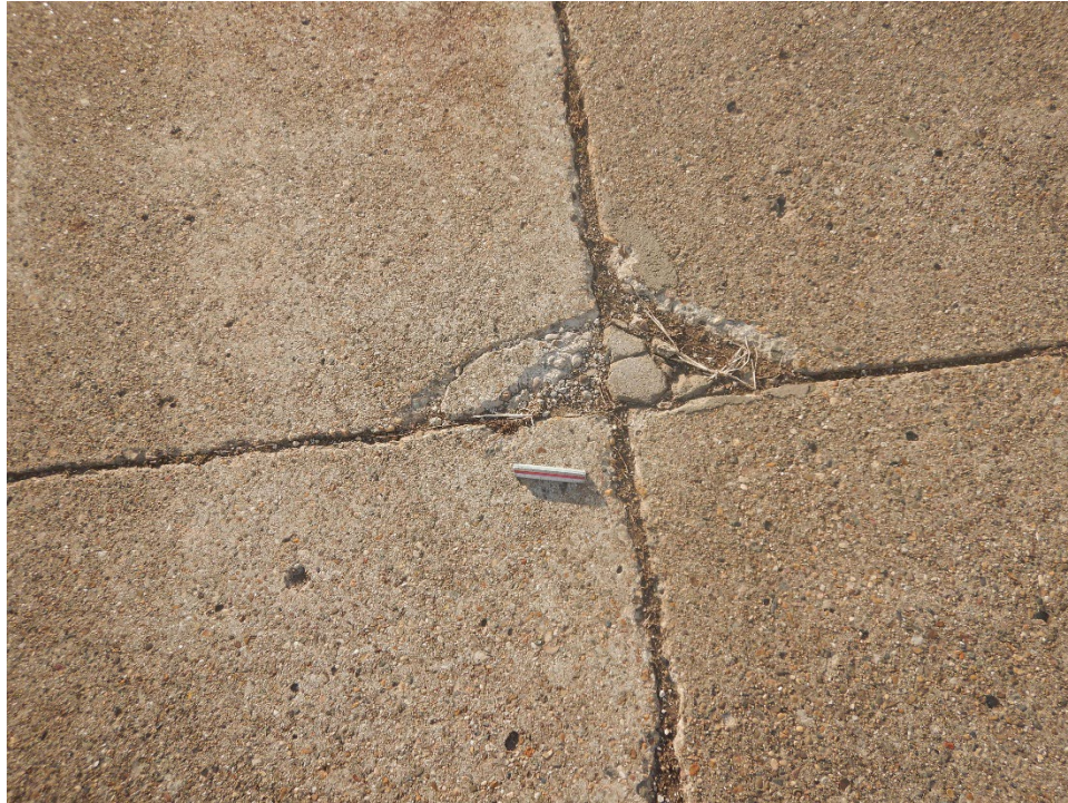
TH01OK-01. Corner Spalling (Sample Unit No. 01).
