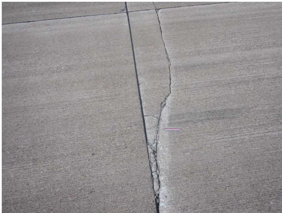
R13OK-01. LTD Cracking (Additional Sample Unit No. 66).
