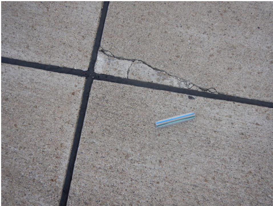
T05OK-01. Corner Spalling (Sample Unit No. 09).
