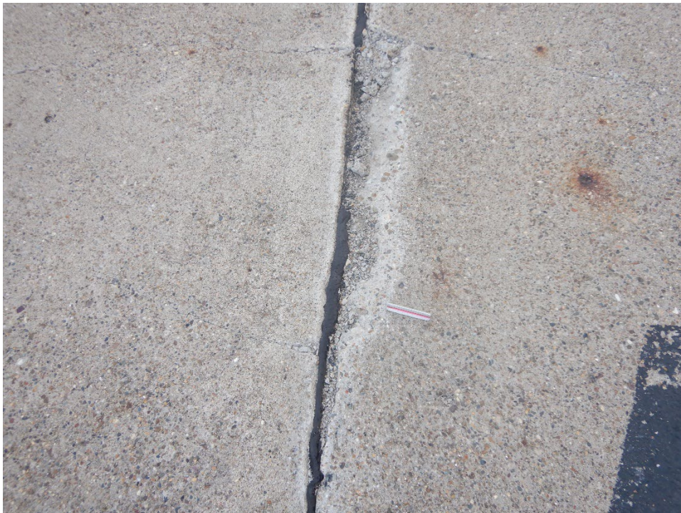
R04OK-01. Joint Spalling (Sample Unit No. 04).
