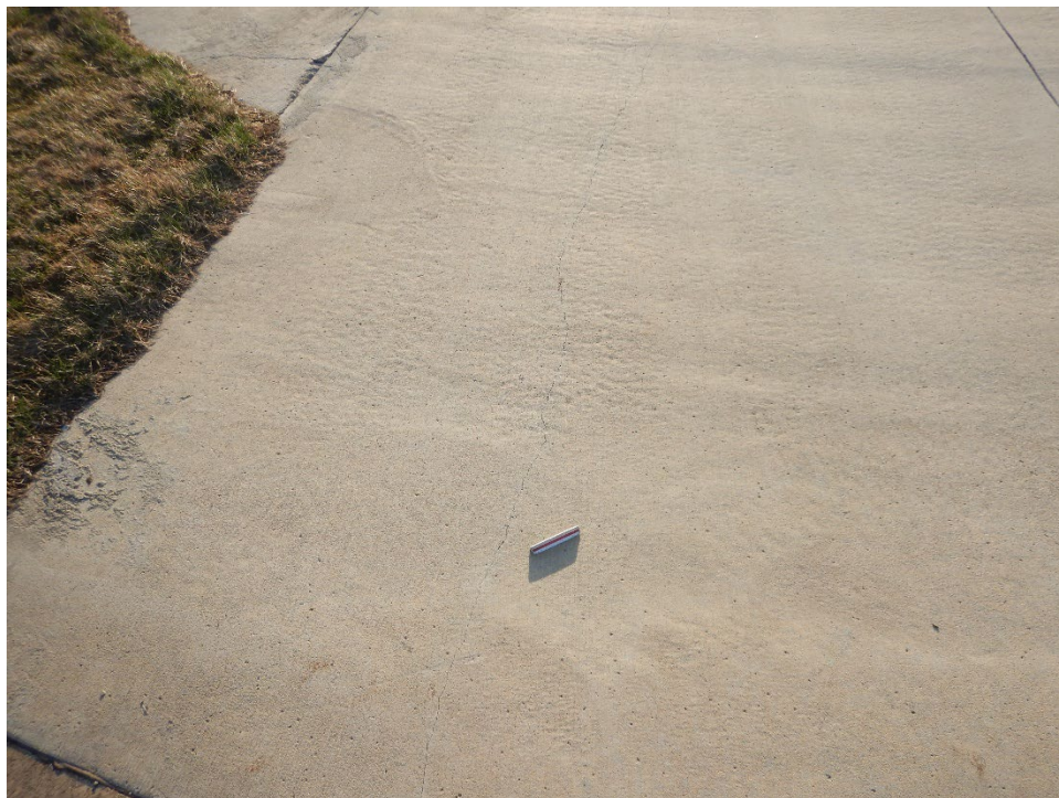
T01OA-01. LTD Cracking (Sample Unit No. 02).
