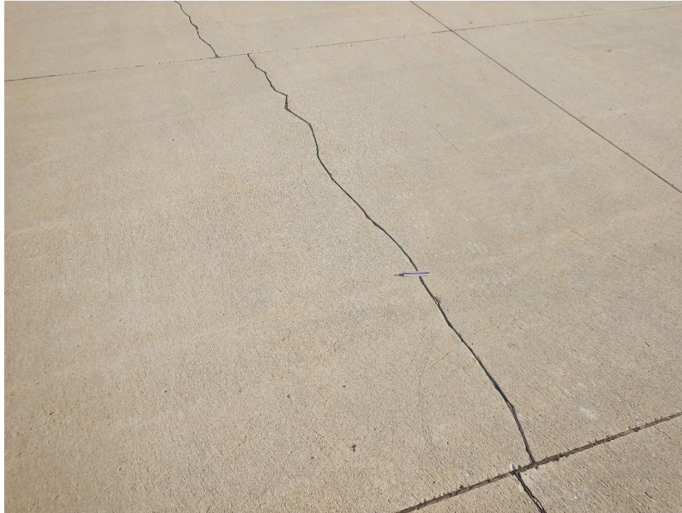
A01OA-02. LTD Cracking (Sample Unit No. 06).
