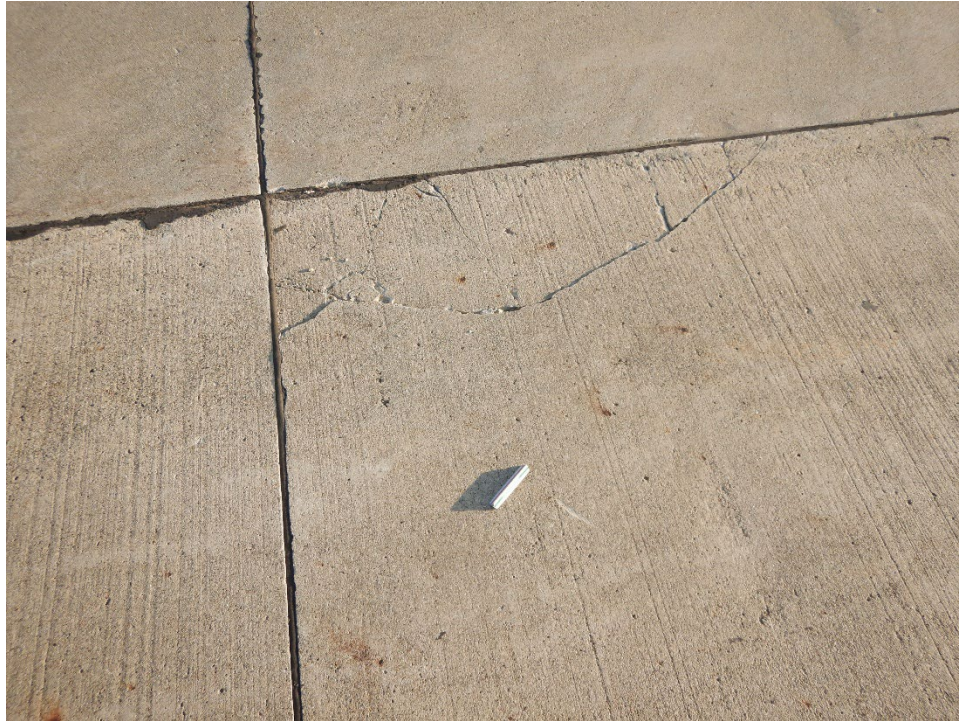
T01OA-01. Corner Spalling (Additional Sample Unit No. 06).
