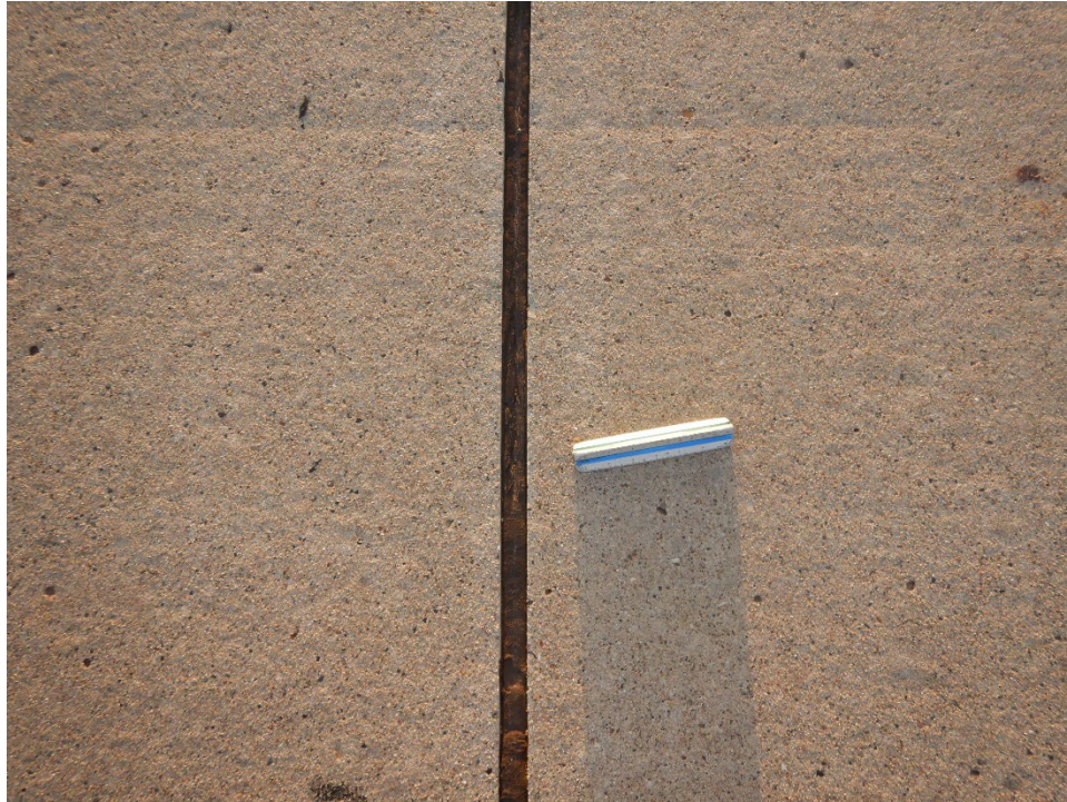
R18OA-01. Joint Seal Damage (Sample Unit No. 75).
