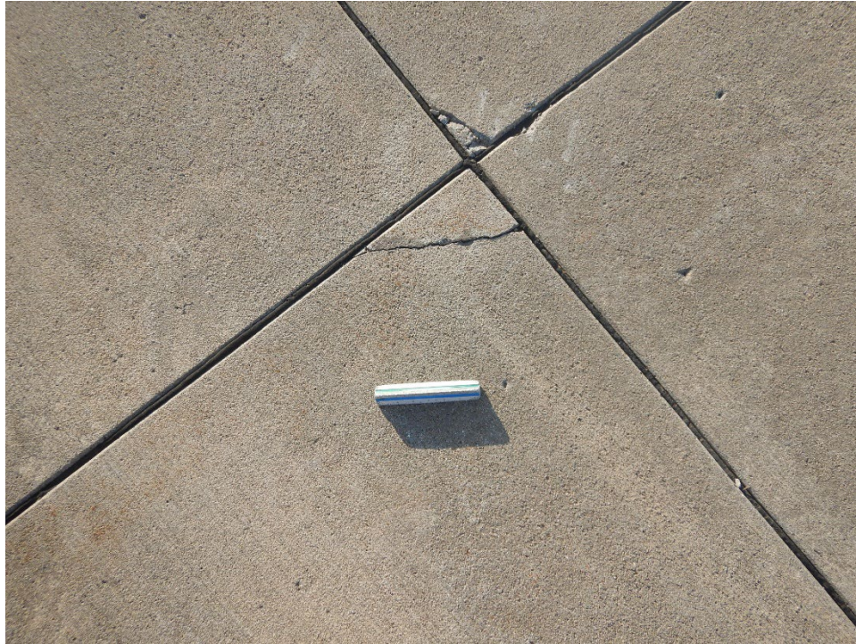
TH01OA-01. Corner Spalling (Sample Unit No. 02).
