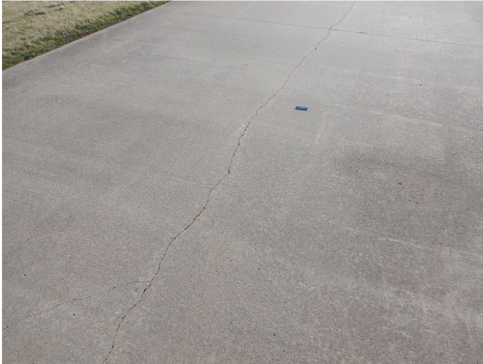
TH02OA-01. LTD Cracking (Sample Unit No. 01).
