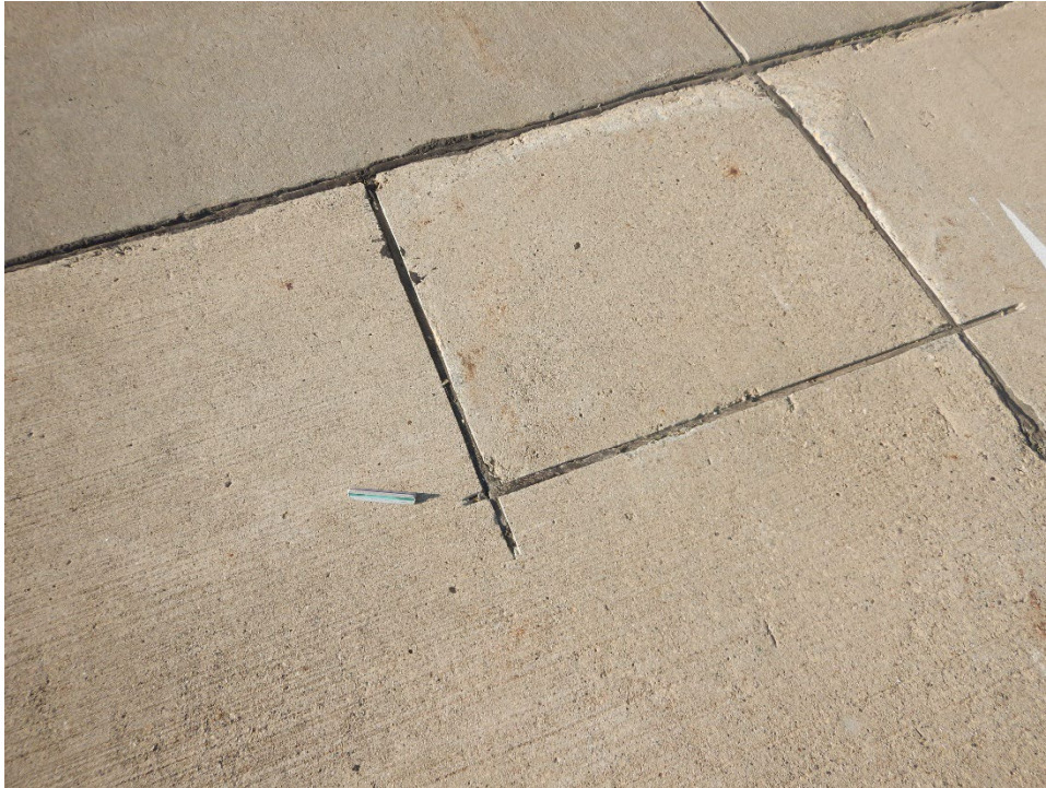
A01OA-01. Large Patching (Sample Unit No. 05).
