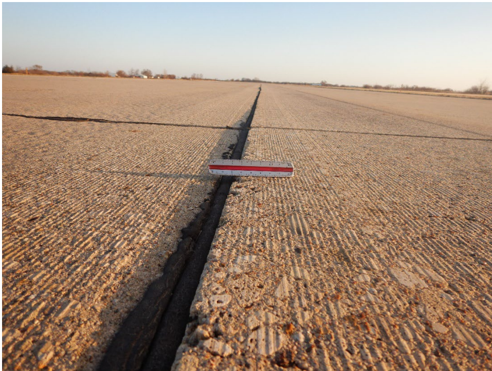
R18OA-01. Faulting (Sample Unit No. 57).
