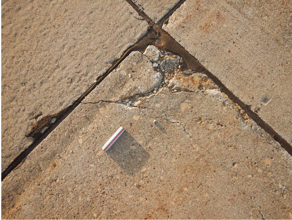
R18OA-01. Corner Spalling (Sample Unit No. 39).
