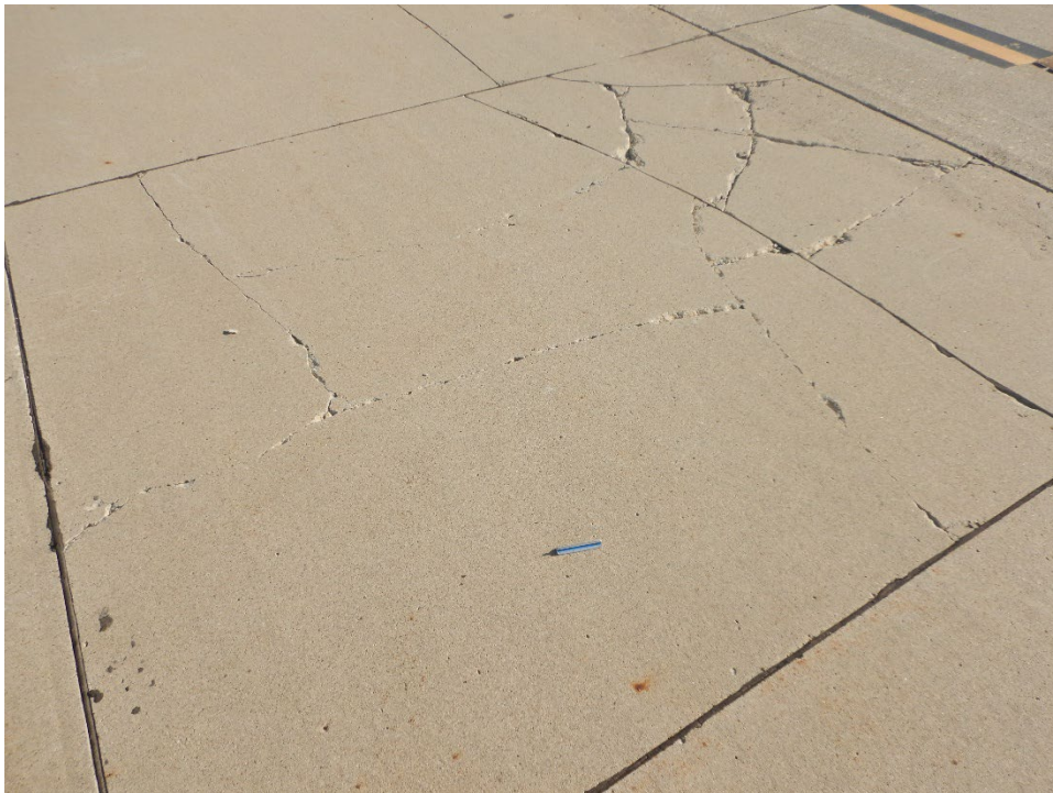
A01OA-01. Shattered Slab (Sample Unit No. 01).
