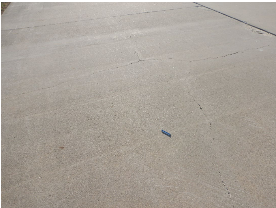
TH02OA-01. Shattered Slab (Sample Unit No. 01).
