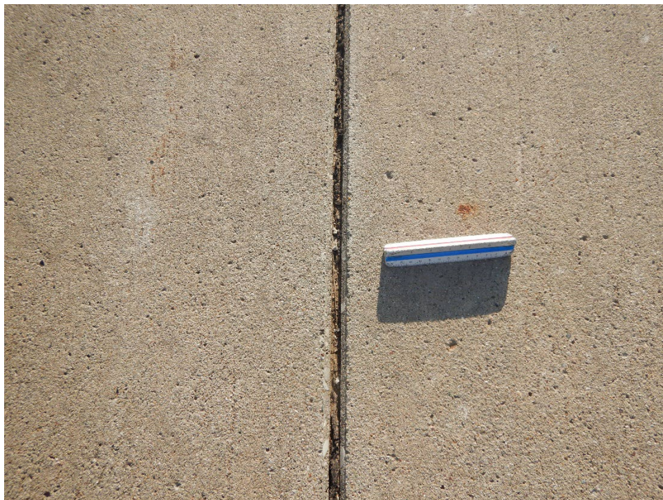
TH01OA-02. Joint Seal Damage (Sample Unit No. 06).
