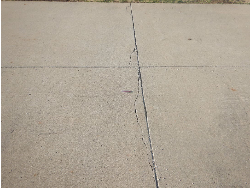
TH01OA-02. Joint Spalling (Additional Sample Unit No. 07).
