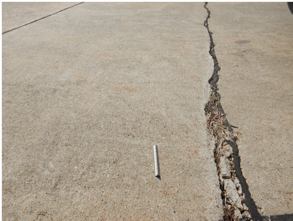
T02OS-02. LTD Cracking (Sample Unit No. 01) (1).
