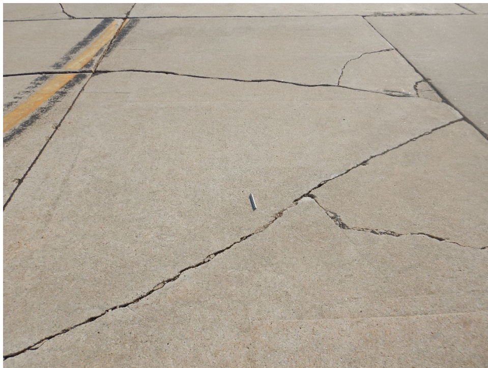
A01OS-02. Shattered Slab (Sample Unit No. 02).
