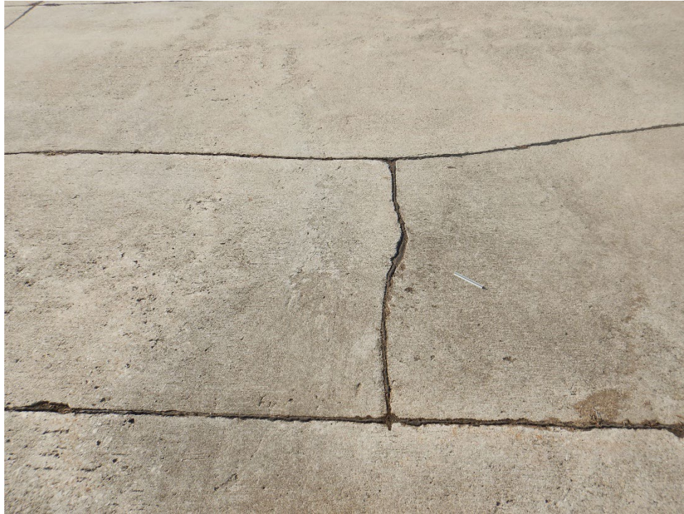
A01OS-01. LTD Cracking (Sample Unit No. 01).
