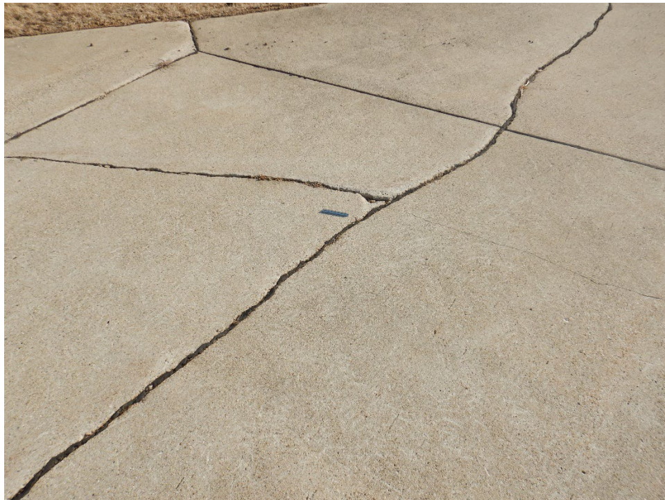
T01OS-01. Shattered Slab (Sample Unit No. 01).
