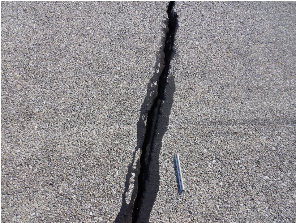
R17OS-01. L&T Cracking (Sample Unit No. 04).
