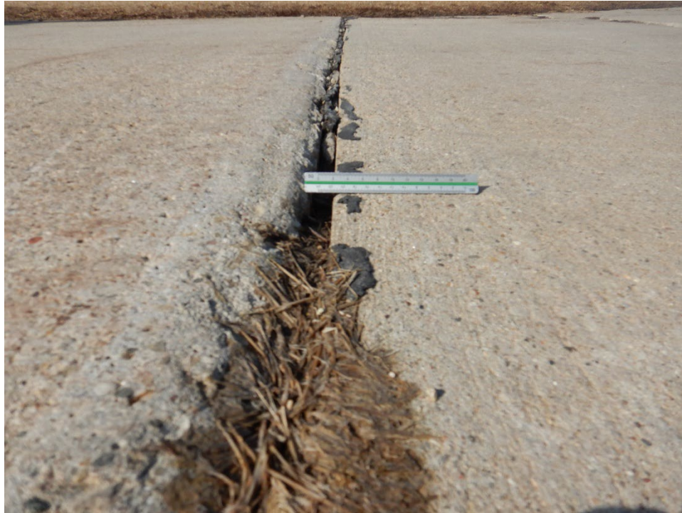
T02OS-02. Faulting (Sample Unit No. 03).
