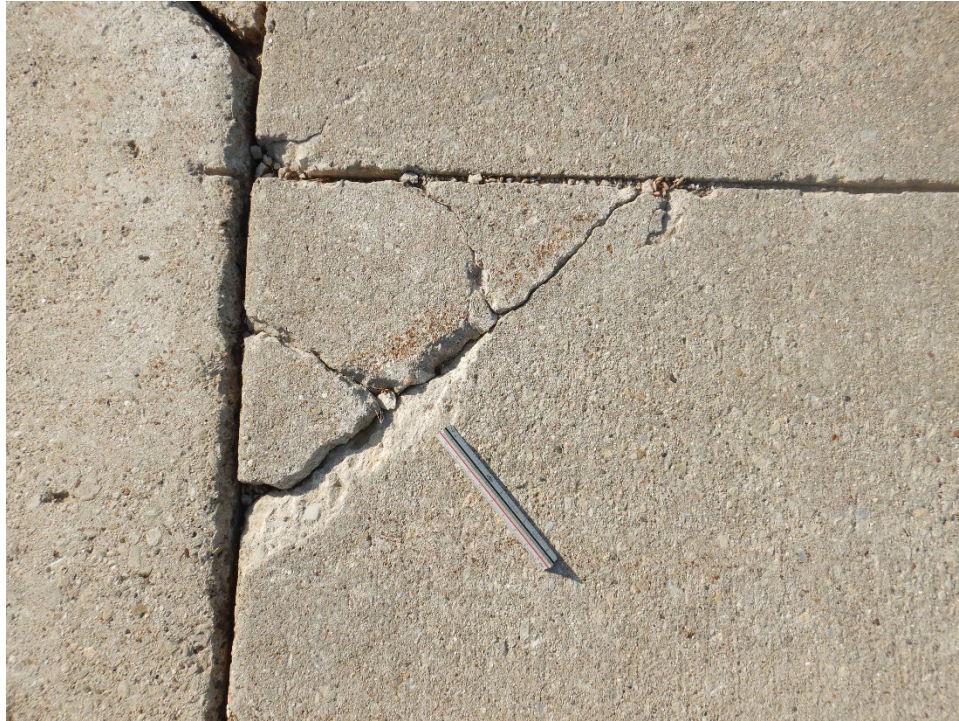
A01OS-02. Corner Spalling (Sample Unit No. 02).
