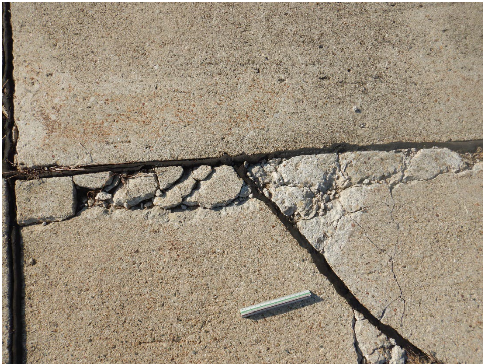
A01OS-01. Joint Spalling (Sample Unit No. 01).
