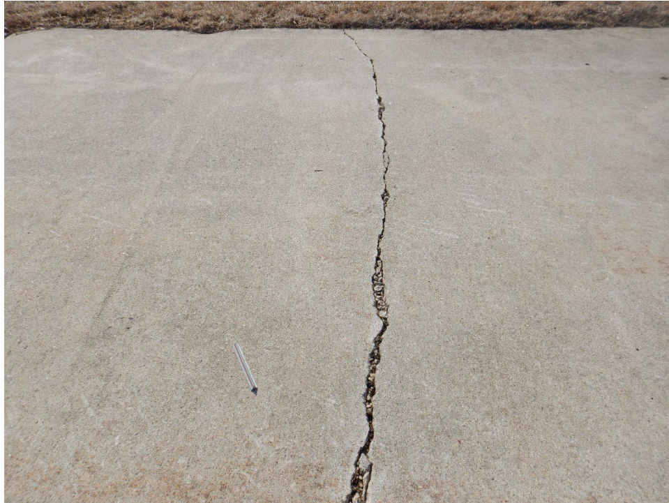
T02OS-02. LTD Cracking (Sample Unit No. 01) (2).
