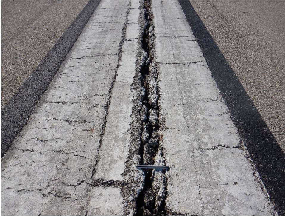
R17OS-01. L&T Cracking (Sample Unit No. 20).
