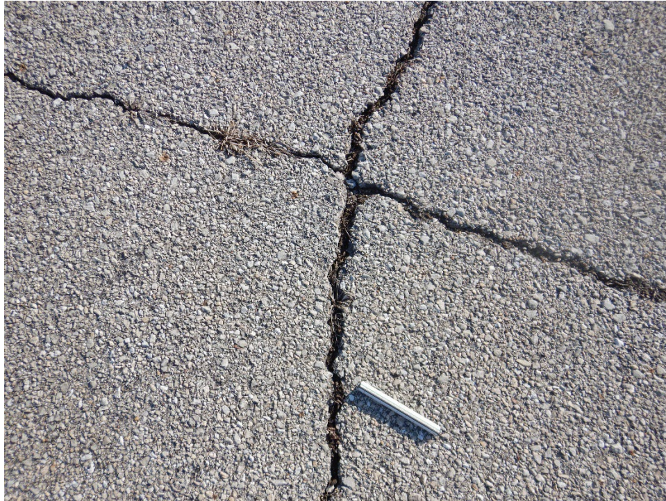
R17OS-02. L&T Cracking (Sample Unit No. 04).
