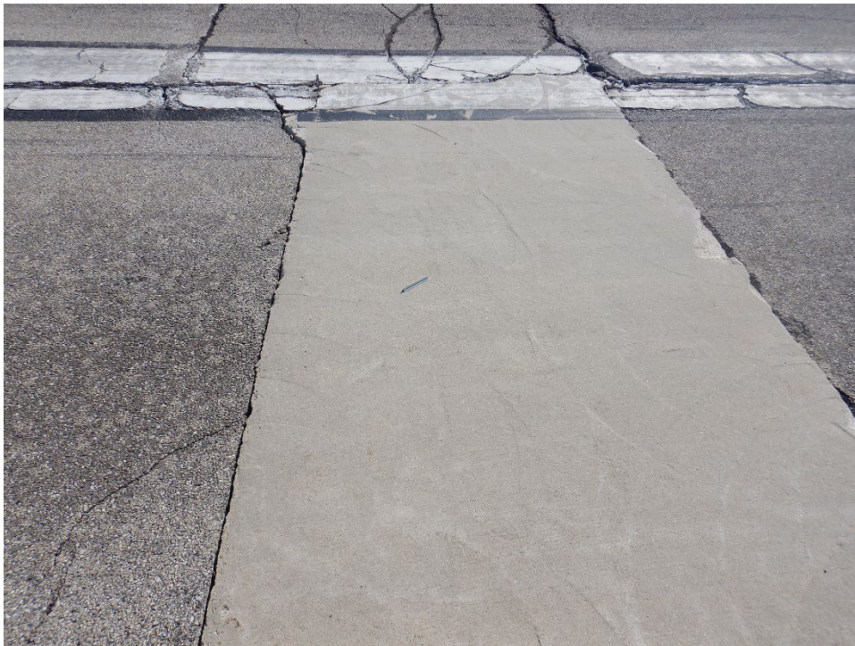
R17OS-01. Patching (Sample Unit No. 04) (1).
