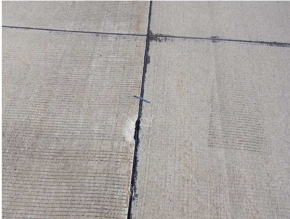
R13OE-01. Joint Spalling (Sample Unit No. 98).
