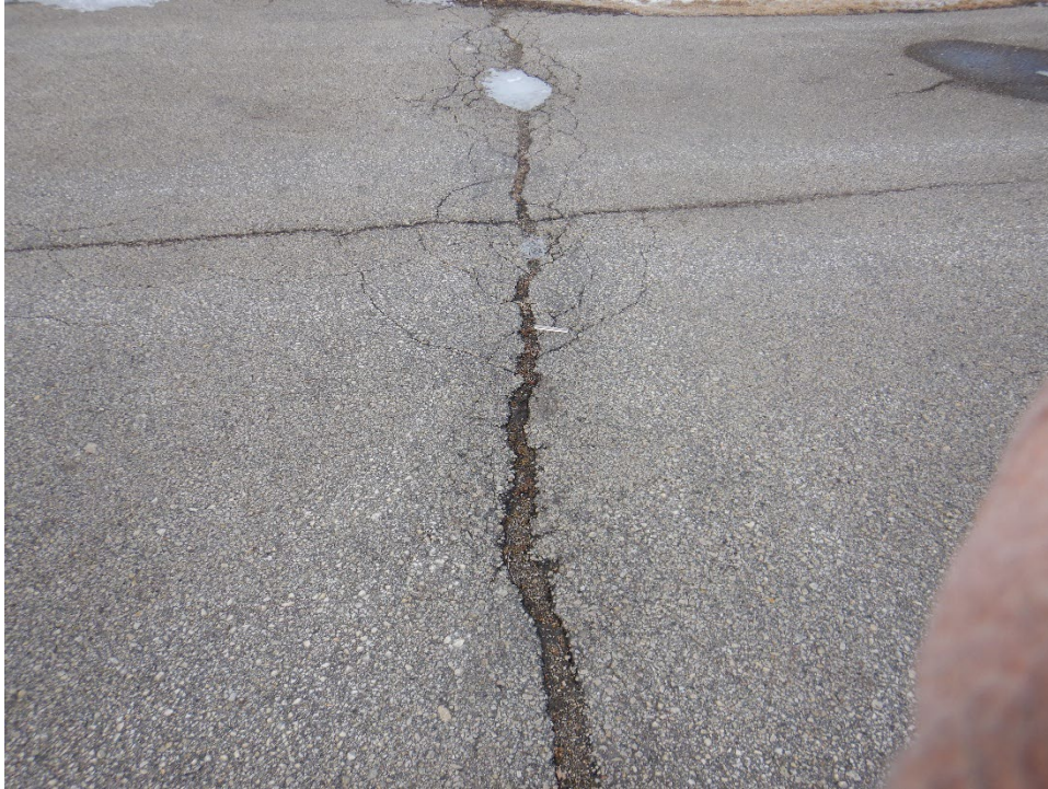
TH01OE-02. Alligator Cracking (Sample Unit No. 01).
