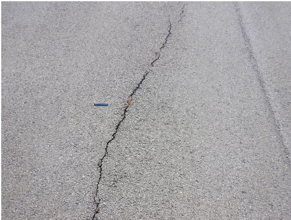
T01OE-02. L&T Cracking (Sample Unit No. 01).
