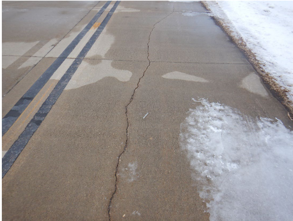
TH01OE-04. LTD Cracking (Sample Unit No. 03).
