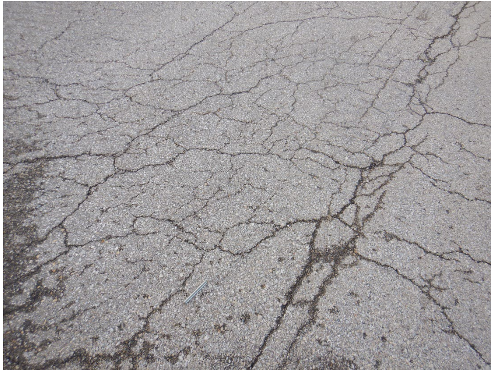
TH01OE-01. Alligator Cracking (Sample Unit No. 01).
