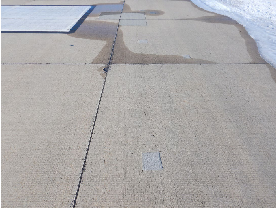
R13OE-01. Small Patching (Additional Sample Unit No. 96).
