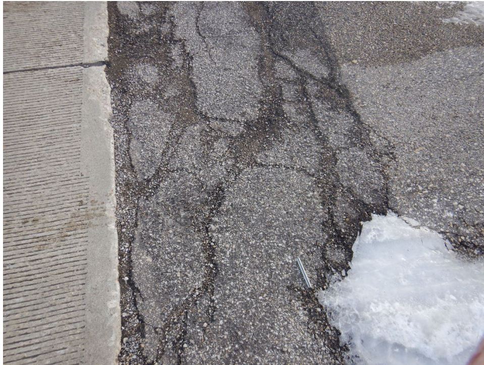
TH01OE-02. Patching (Sample Unit No. 02).
