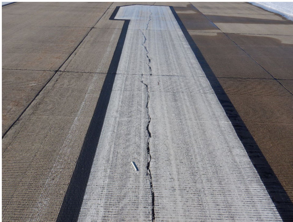
R13OE-01. LTD Cracking (Additional Sample Unit No. 97).
