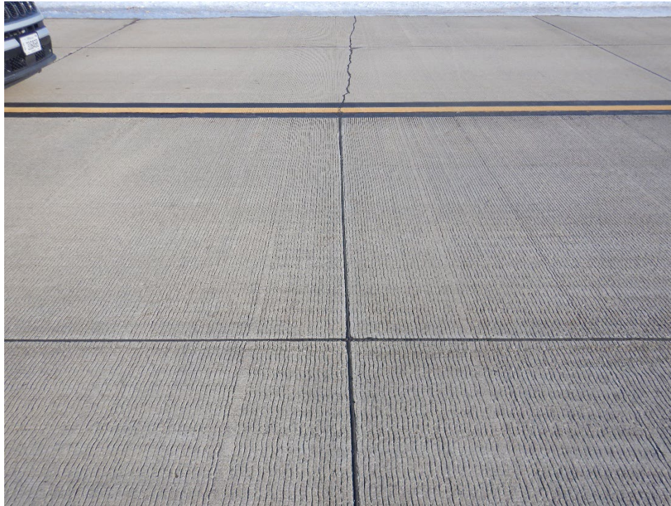
T01OE-01. LTD Cracking (Sample Unit No. 07).
