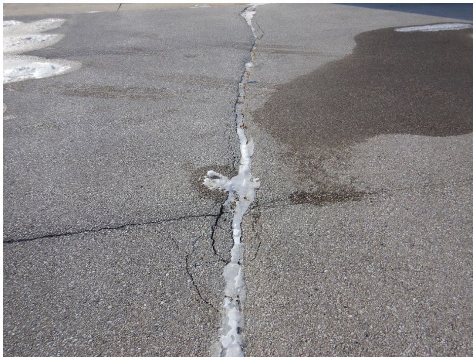
TH01OE-01. L&T Cracking (Sample Unit No. 02).
