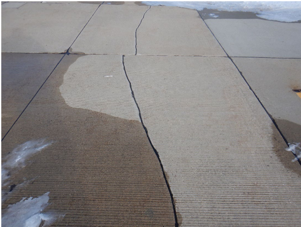
A01OE-01. LTD Cracking (Sample Unit No. 19).
