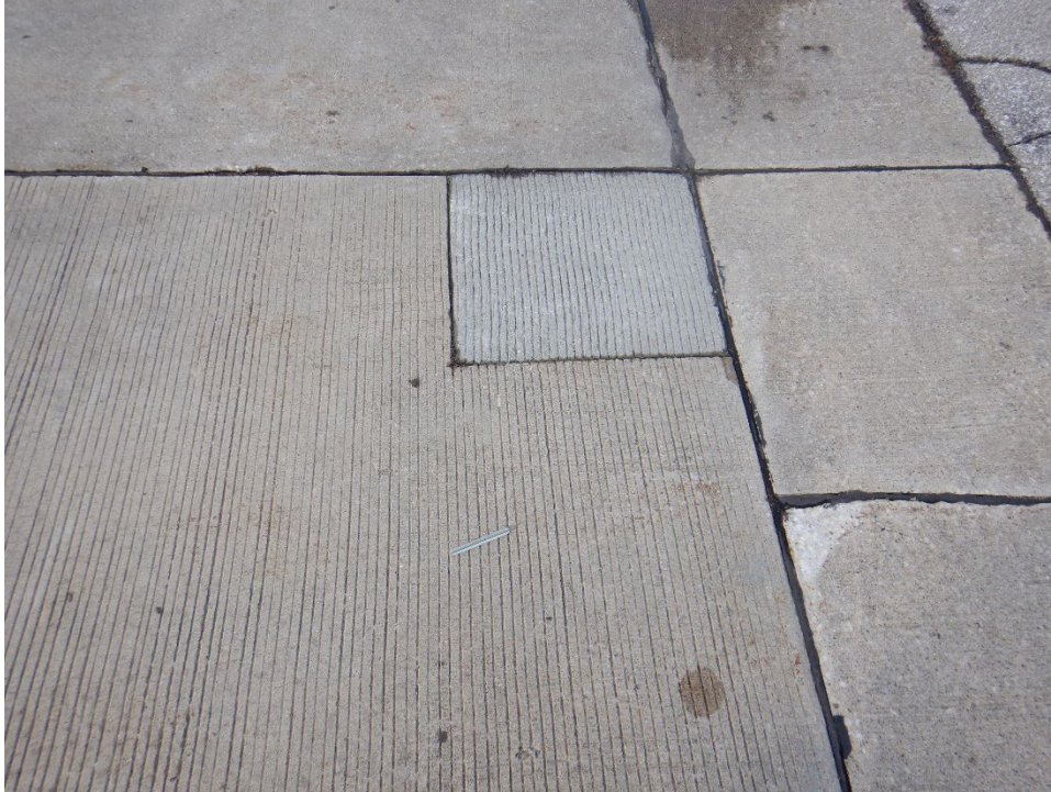
A01OE-01. Small Patching (Sample Unit No. 19).
