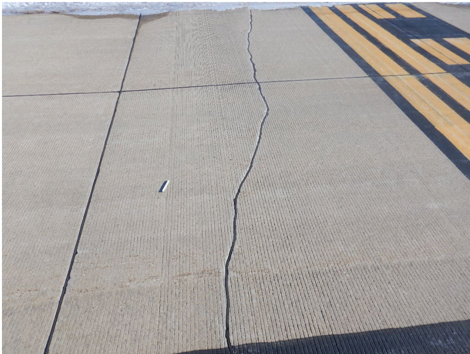
T01OE-01. LTD Cracking (Additional Sample Unit No. 013).
