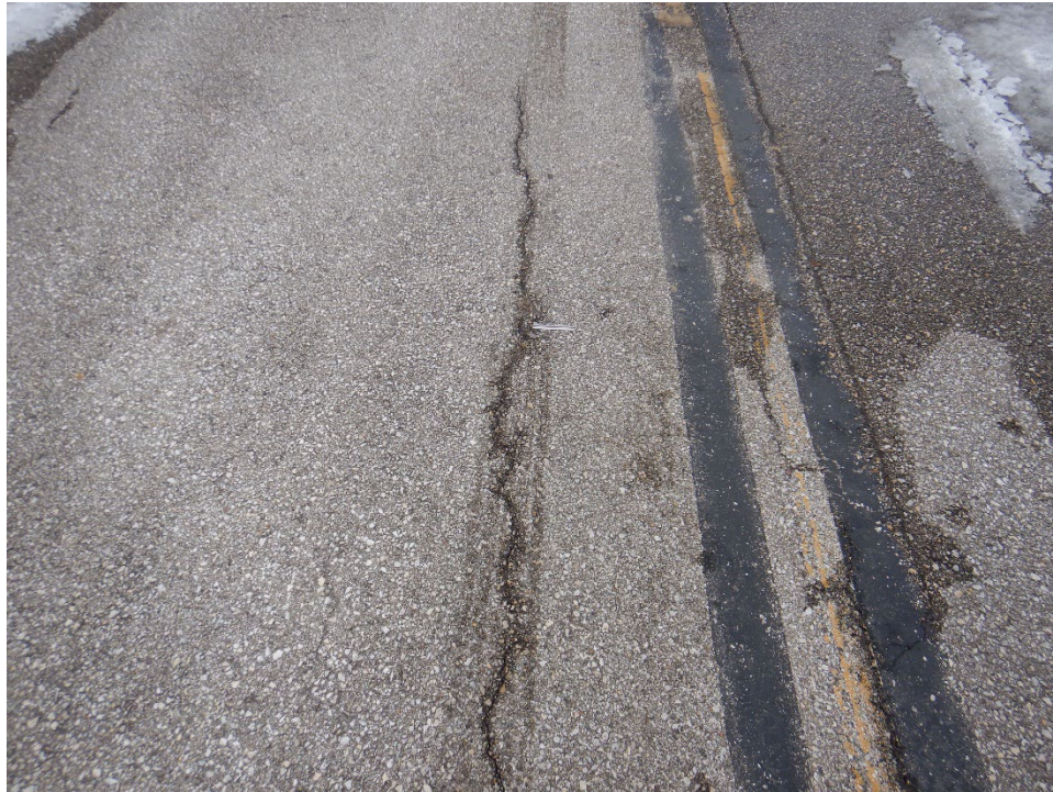
TH01OE-03. L&T Cracking (Sample Unit No. 02).
