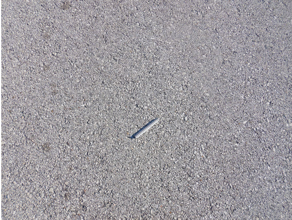
T01OE-02. Weathering (Sample Unit No. 01).
