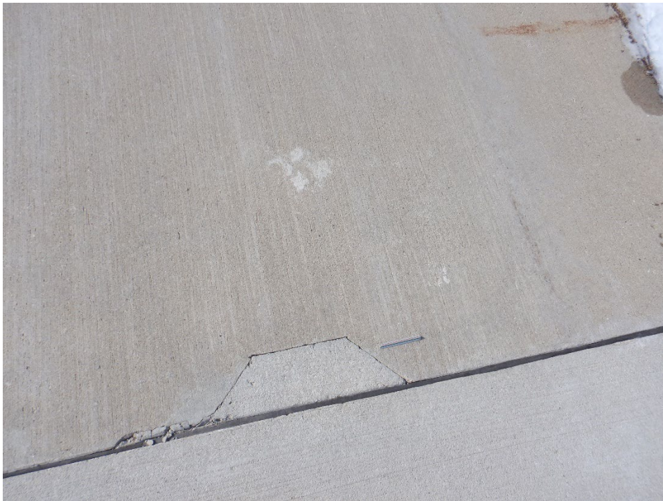
TH01CC-02. Small Patching (Sample Unit No. 01).
