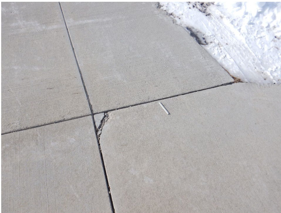
T03CC-01. Corner Spalling (Sample Unit No. 02).
