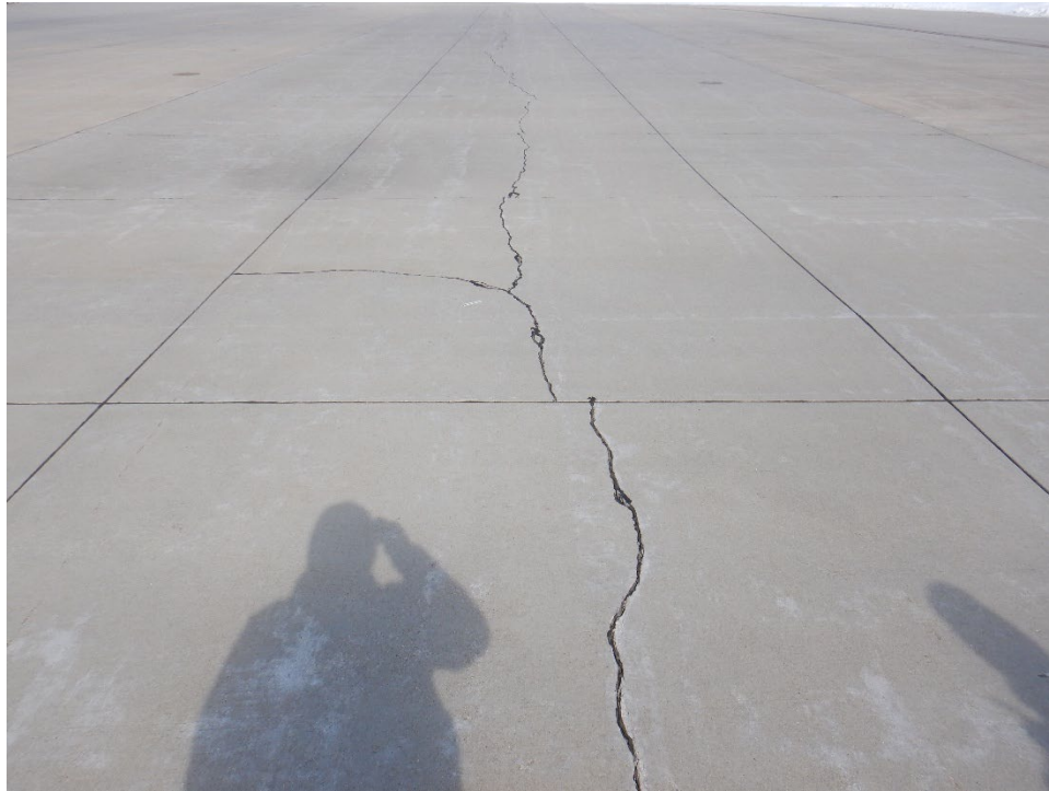
A04CC-01. LTD Cracking (Sample Unit No. 14).
