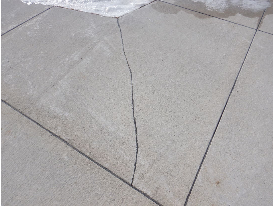
T03CC-01. LTD Cracking (Sample Unit No. 25).
