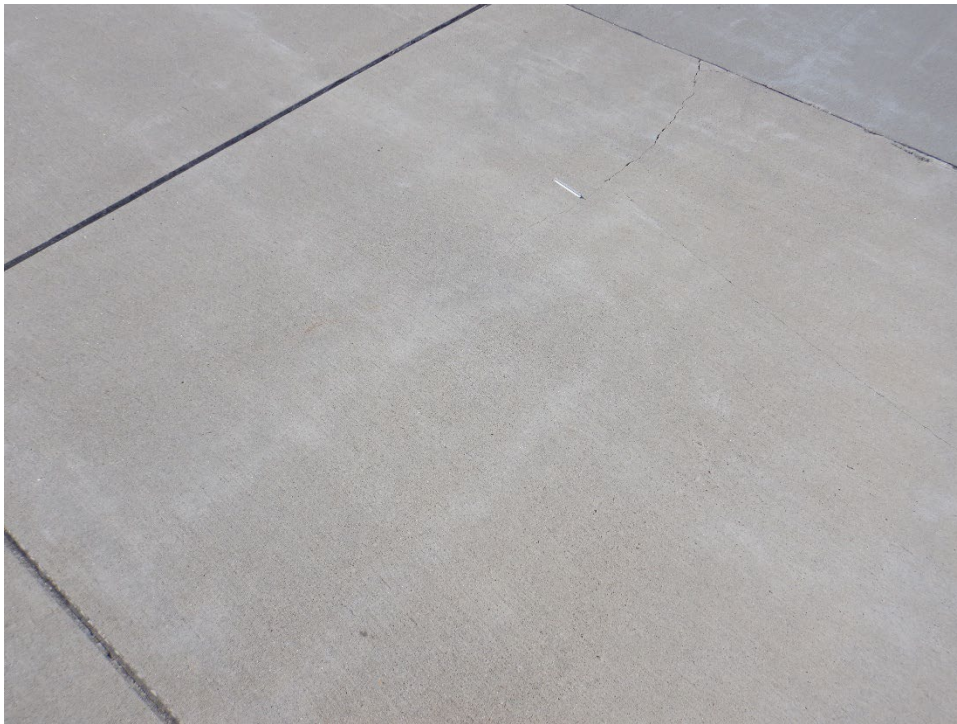
A03CC-01. LTD Cracking (Sample Unit No. 07).
