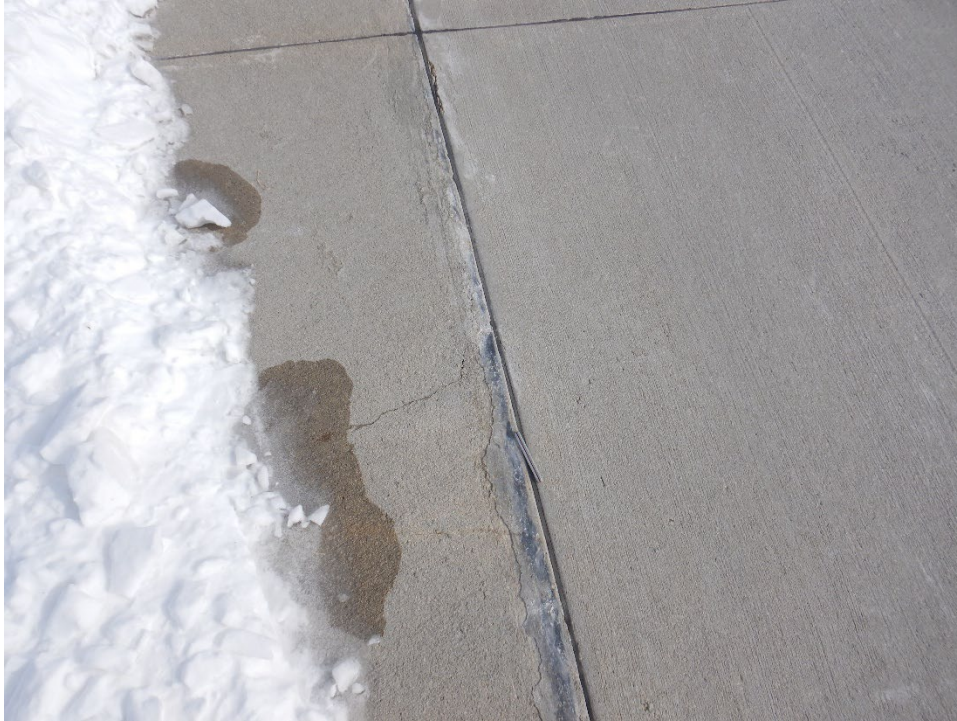
TA1CC-01. Shrinkage Cracking (Sample Unit No. 02).
