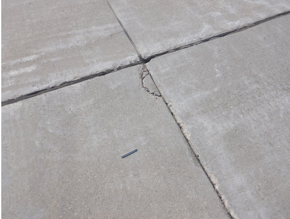
A01CC-01. Joint Spalling (Sample Unit No. 01).
