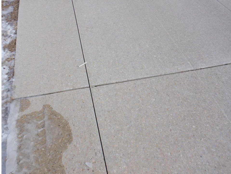
TA2CC-01. Joint Seal Damage (Sample Unit No. 09).
