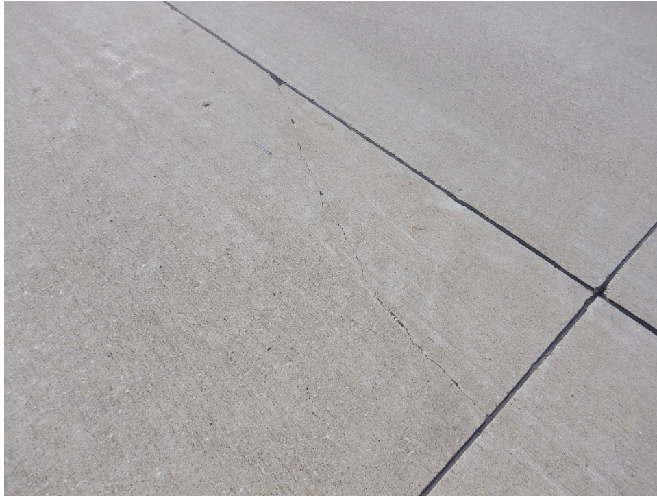
R12CC-01. Corner Break (Sample Unit No. 20).
