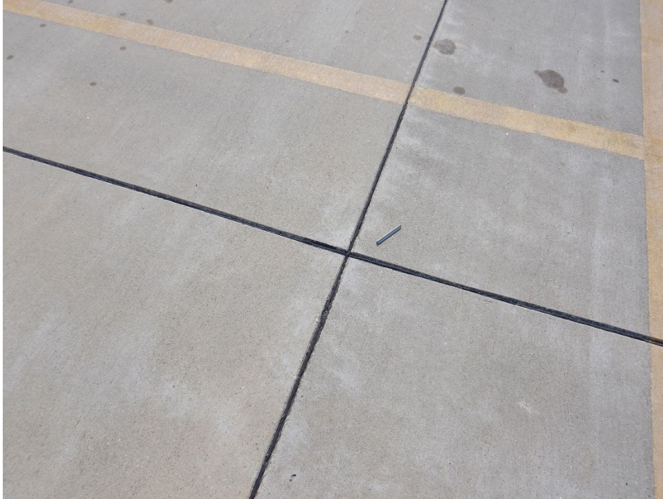
A03CC-01. Joint Seal Damage (Sample Unit No. 07).
