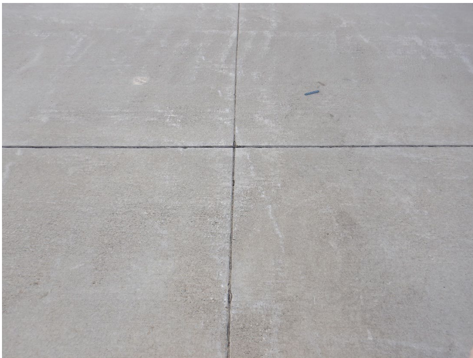
A04CC-01. Joint Seal Damage (Sample Unit No. 10).
