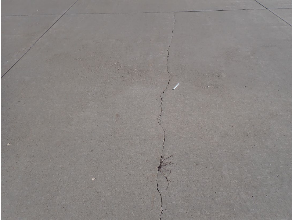
TH02NE-01. LTD Cracking (Sample Unit No. 04).
