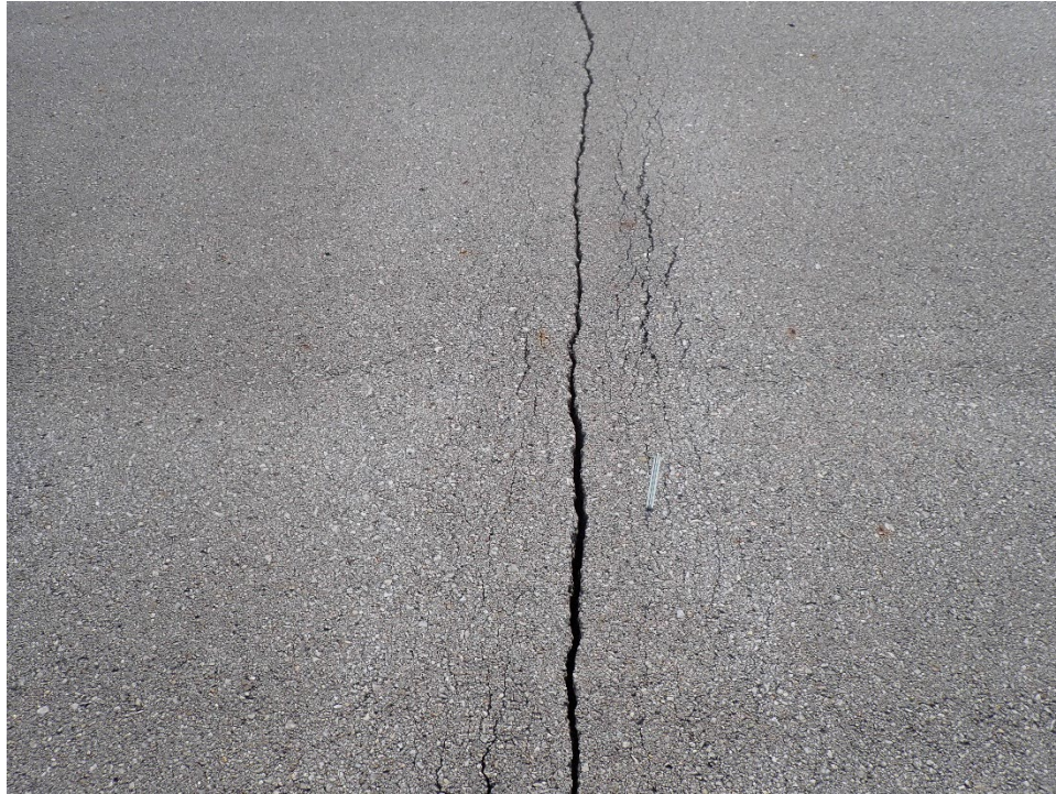
T03NE-01. L&T Cracking (Sample Unit No. 01).
