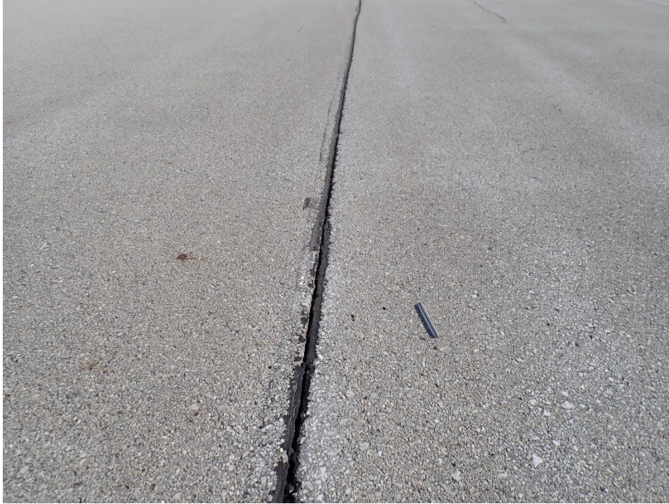
R14NE-02. L&T Cracking (Sample Unit No. 02).
