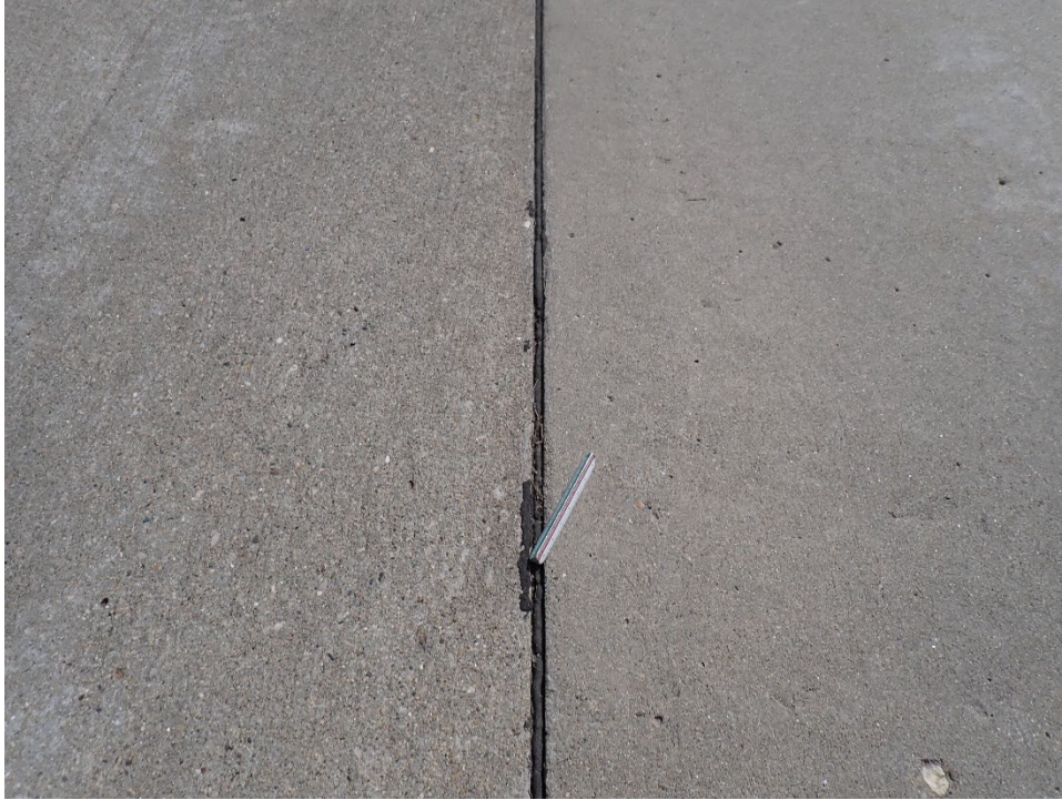
A03NE-01. Joint Seal Damage (Sample Unit No. 15).
