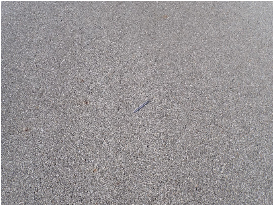
T05NE-01. Weathering (Sample Unit No. 20).
