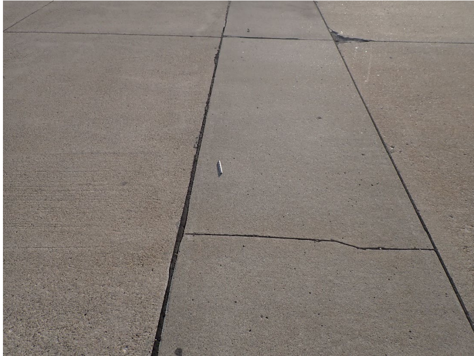
TH01NE-01. Large Patching (Sample Unit No. 03).
