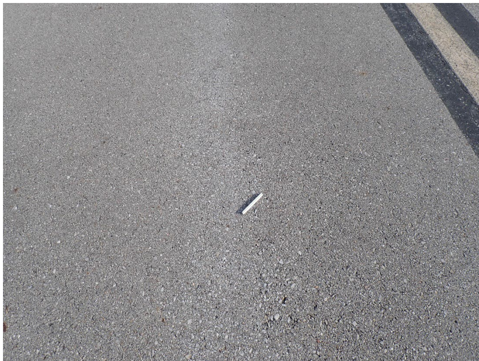
T03NE-01. Weathering (Sample Unit No. 01).
