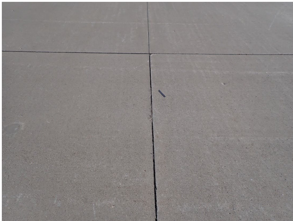
TH02NE-01. Joint Seal Damage (Sample Unit No. 04).
