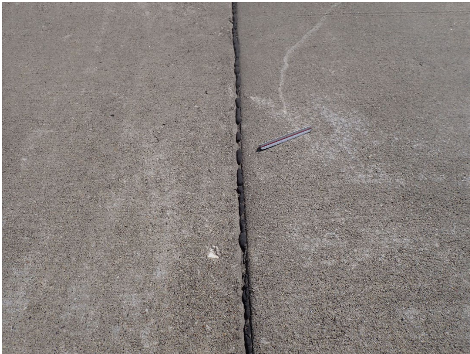
A03NE-02. Joint Seal Damage (Sample Unit No. 10).
