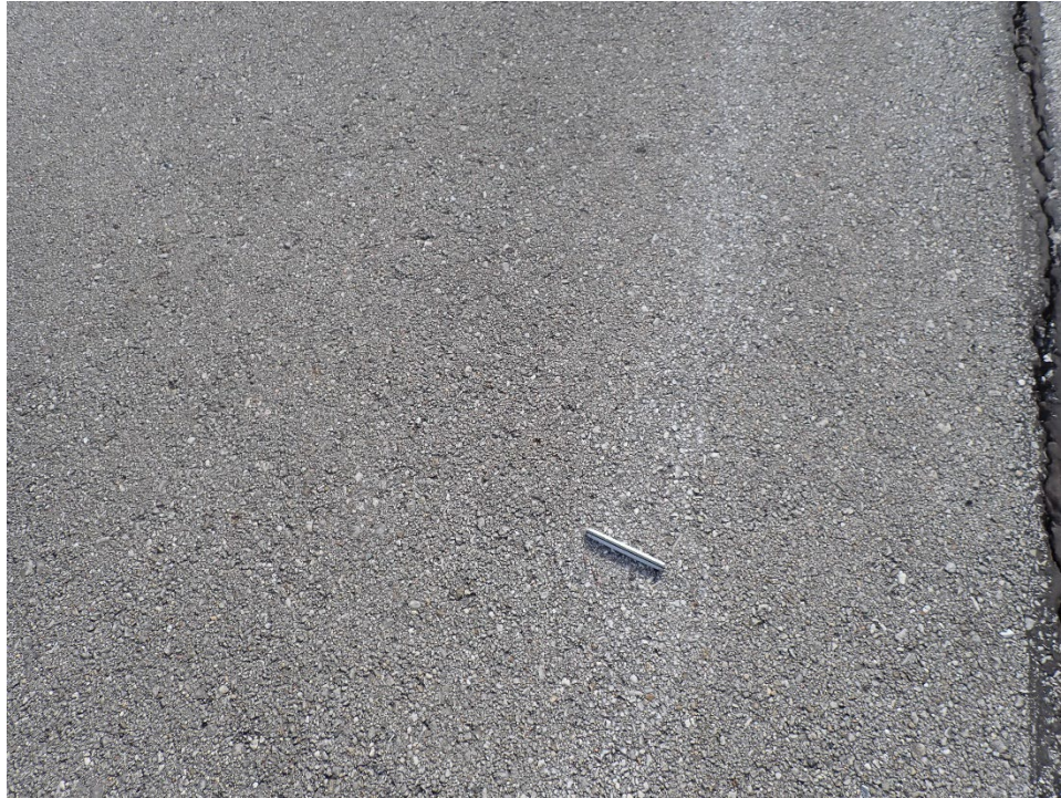
T06NE-01. Weathering (Sample Unit No. 01).
