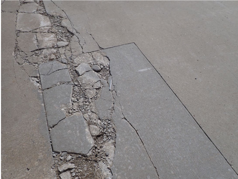
A03NE-01. Large Patching (Additional Sample Unit No. 16).
