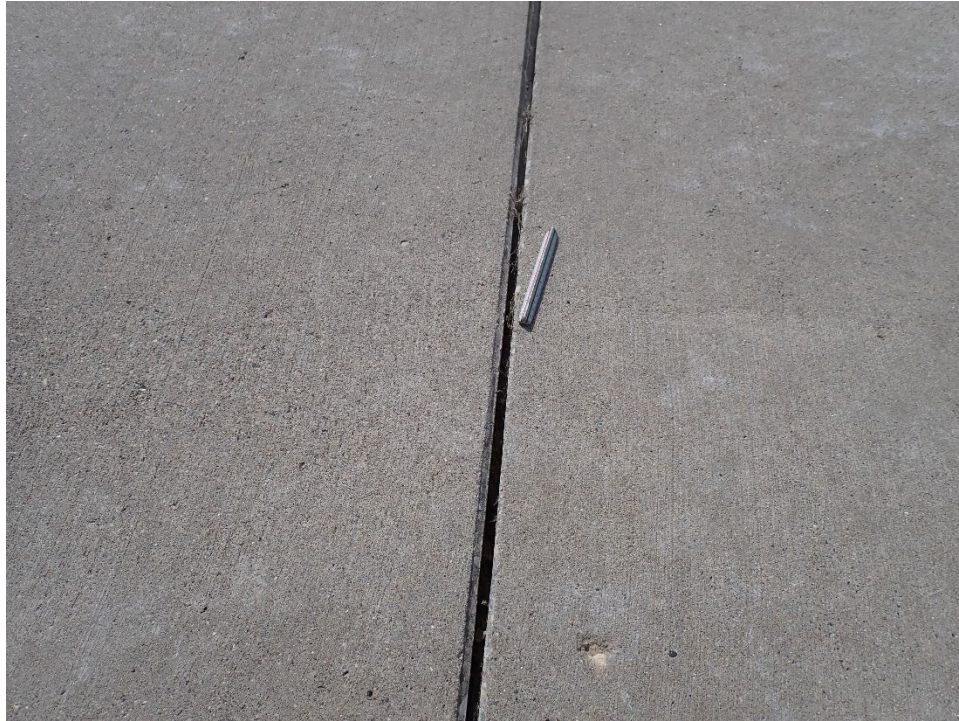
A03NE-03. Joint Seal Damage (Sample Unit No. 10).
