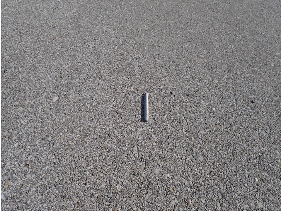
R14NE-03. Weathering (Sample Unit No. 04) (2).
