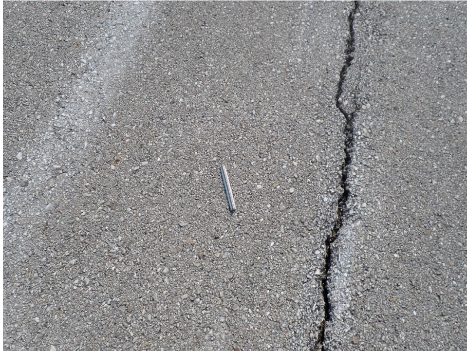
T07NE-01. Weathering (Sample Unit No. 01).
