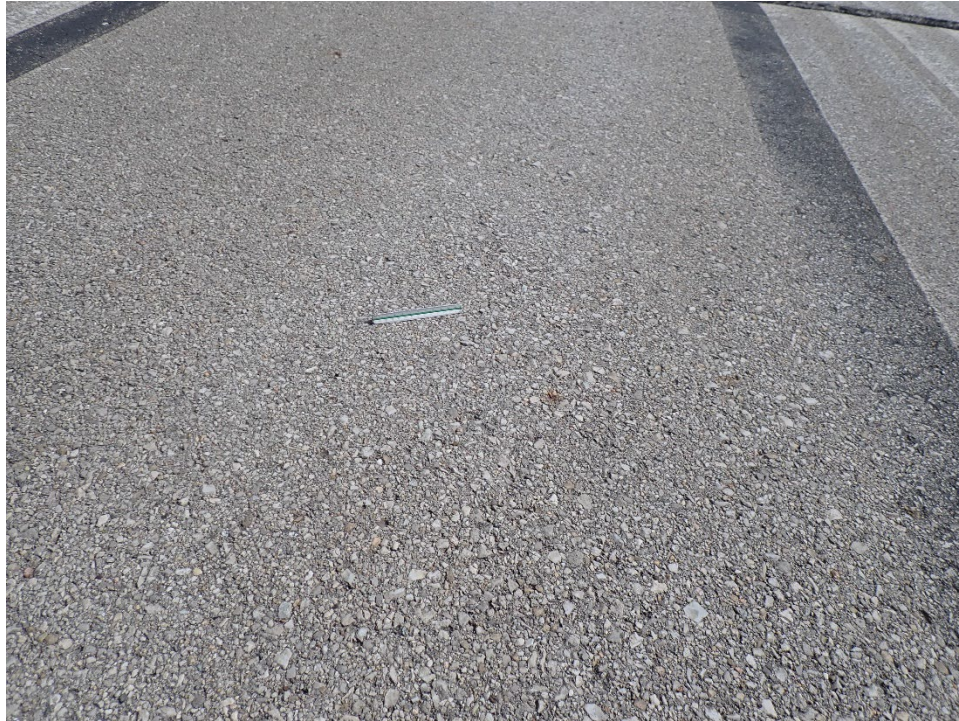
R14NE-01. Weathering (Sample Unit No. 01).
