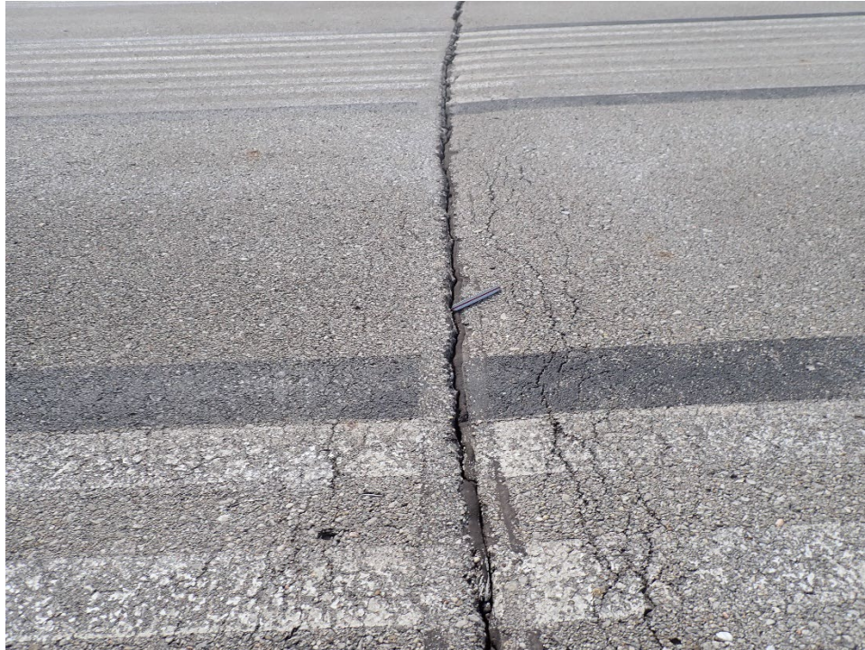
R14NE-01. L&T Cracking (Sample Unit No. 01).
