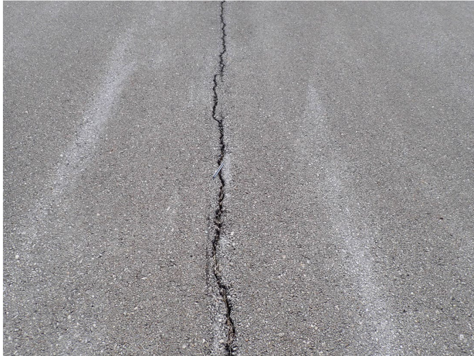
T07NE-01. L&T Cracking (Sample Unit No. 01).
