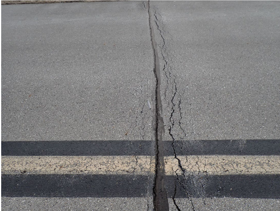
T05NE-01. L&T Cracking (Sample Unit No. 20).
