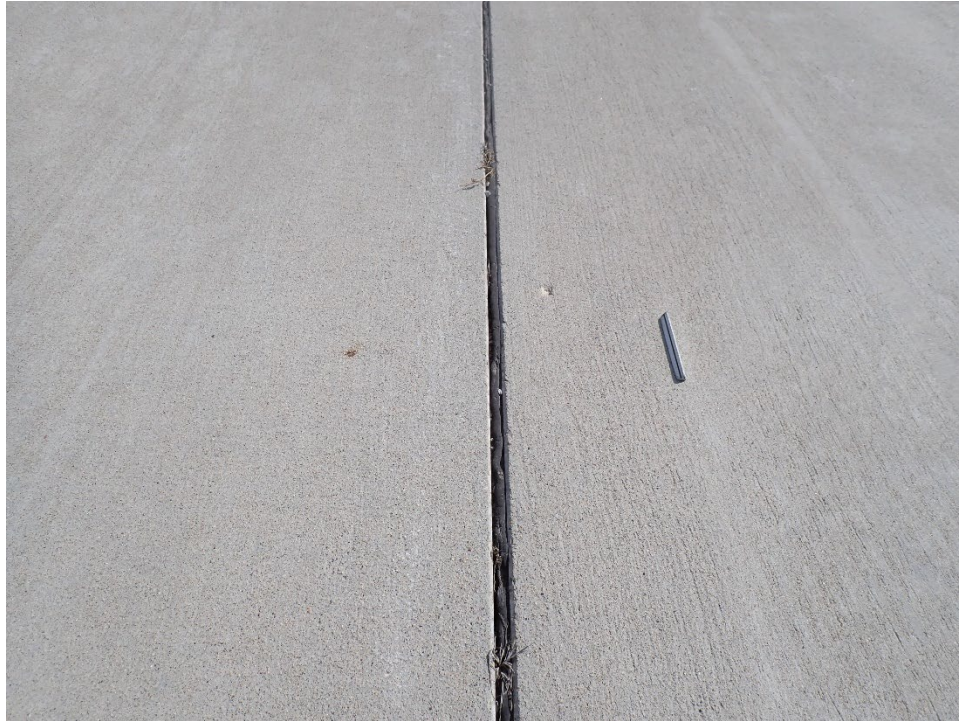
A03NE-04. Joint Seal Damage (Sample Unit No. 03).
