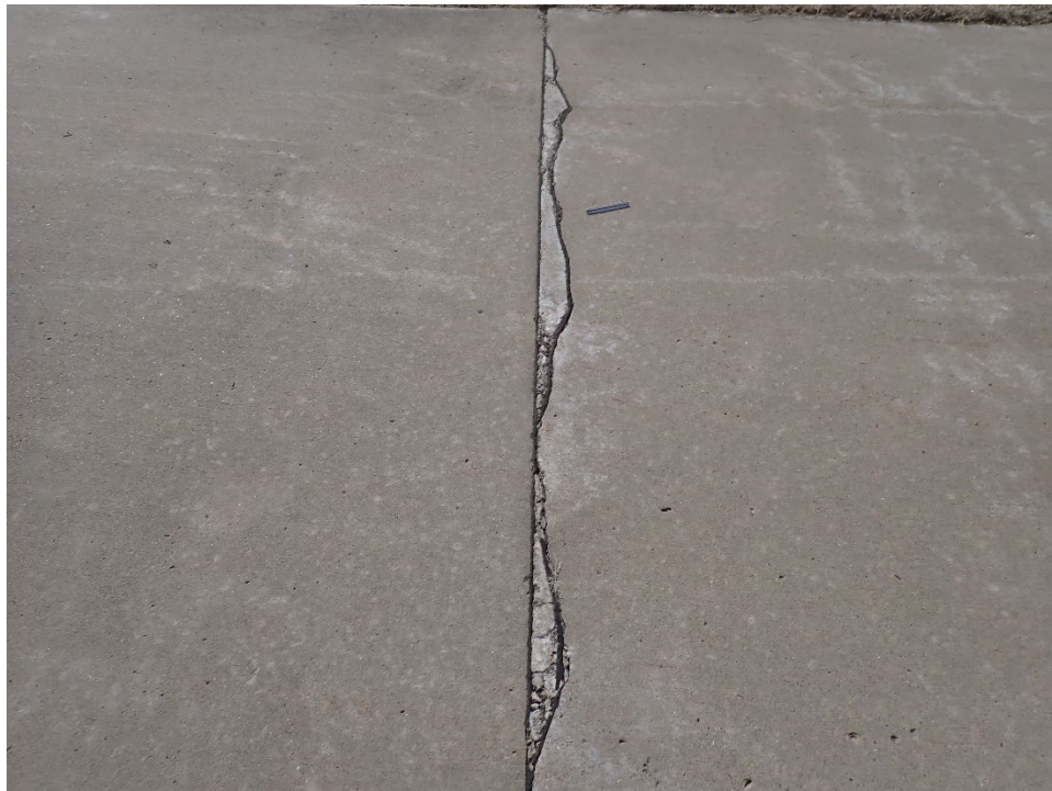
TH03NE-01. Joint Spalling (Sample Unit No. 09).
