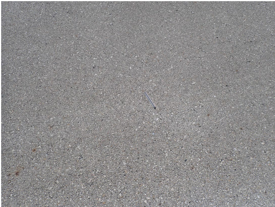
R14NE-02. Weathering (Sample Unit No. 02).
