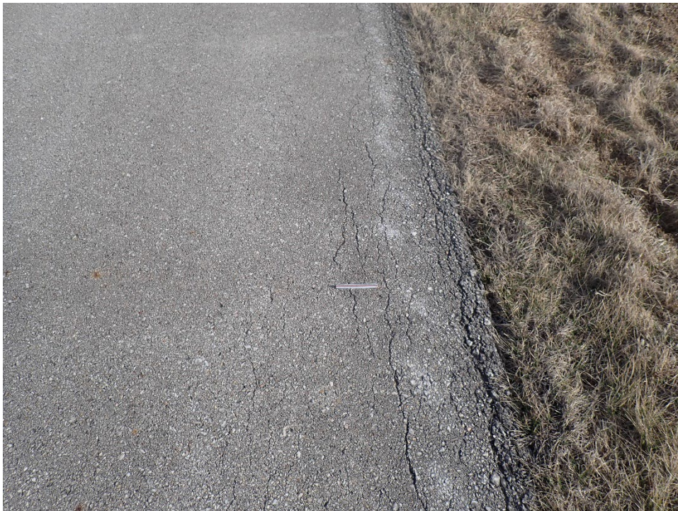
T03NE-01. Alligator Cracking (Sample Unit No. 01).
