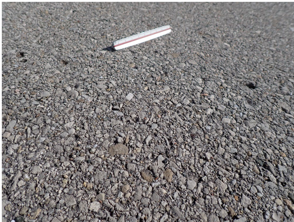
R14NE-03. Weathering (Sample Unit No. 04) (1).
