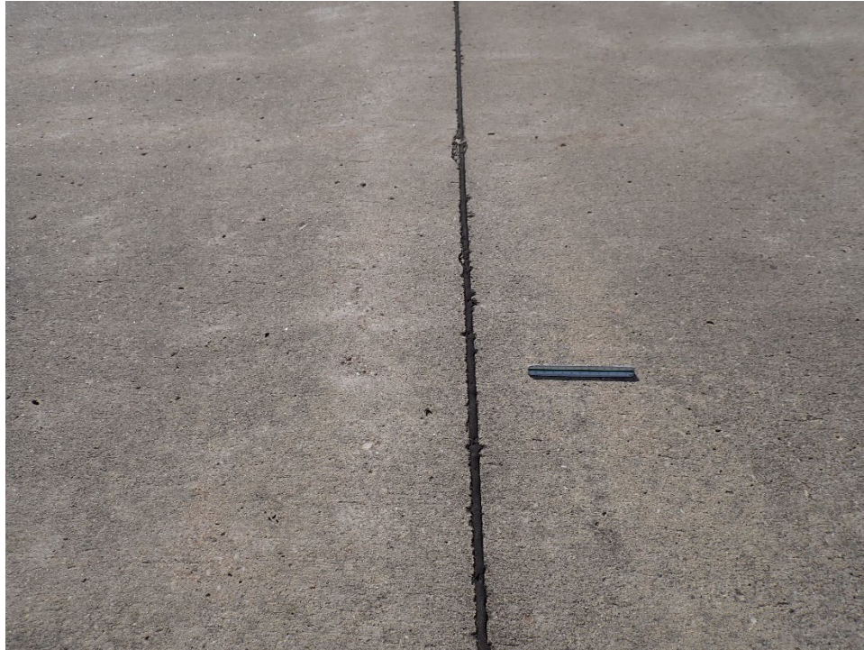
TH03NE-01. Joint Seal Damage (Sample Unit No. 02).
