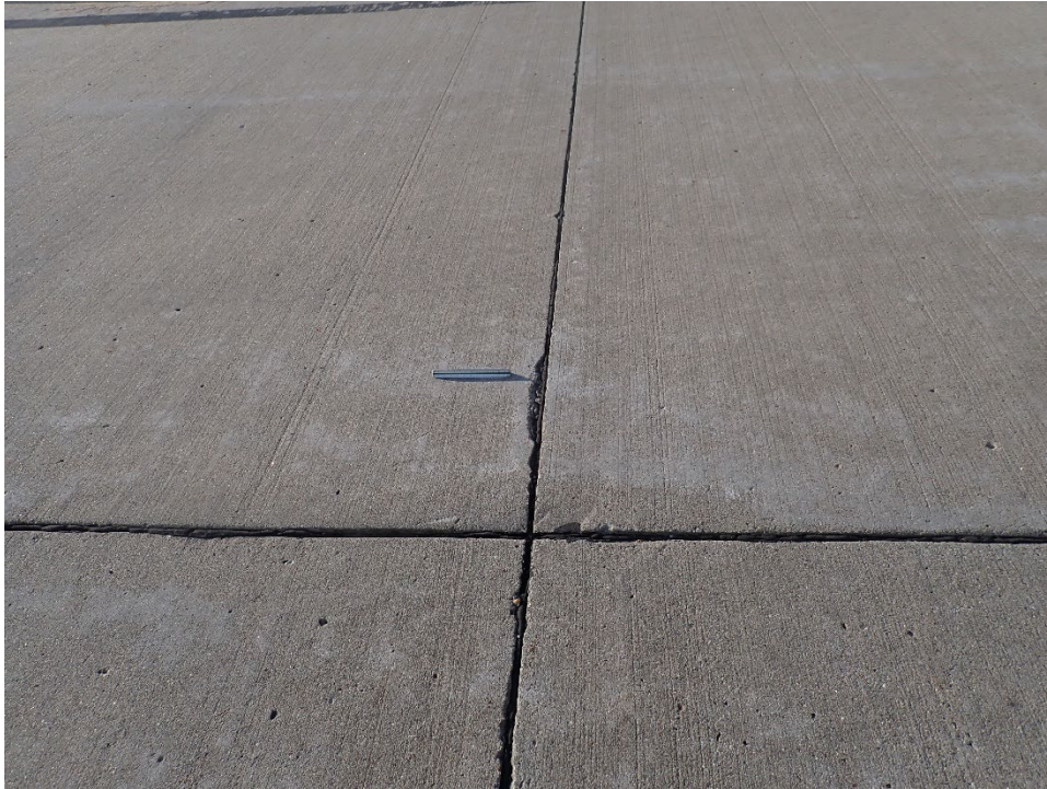
T08NE-01. Joint Seal Damage (Sample Unit No. 01).
