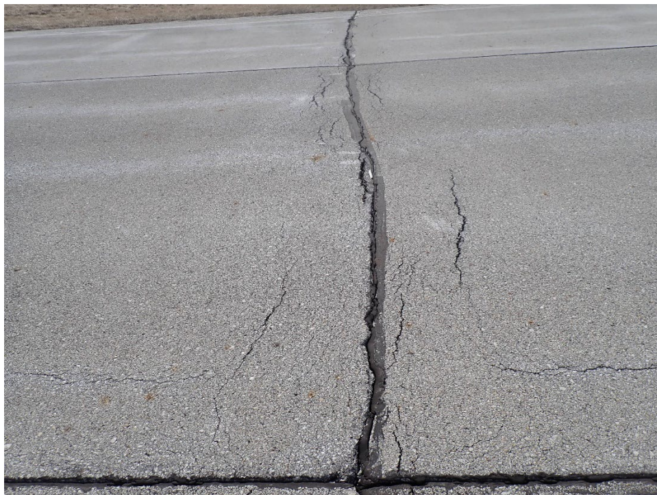
R14NE-01. L&T Cracking (Sample Unit No. 08).
