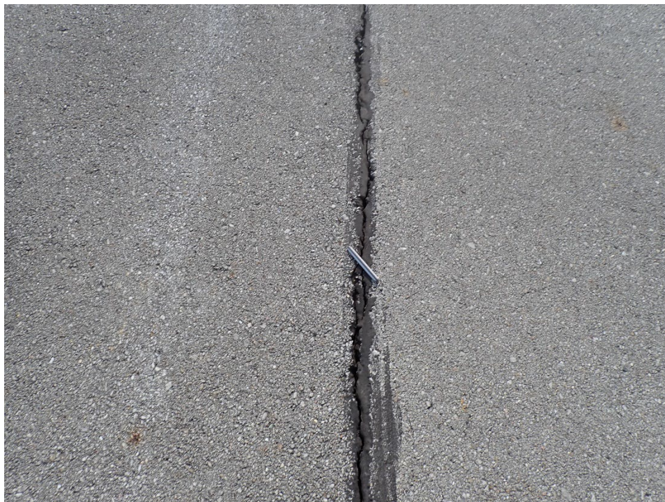
T06NE-01. L&T Cracking (Sample Unit No. 01).
