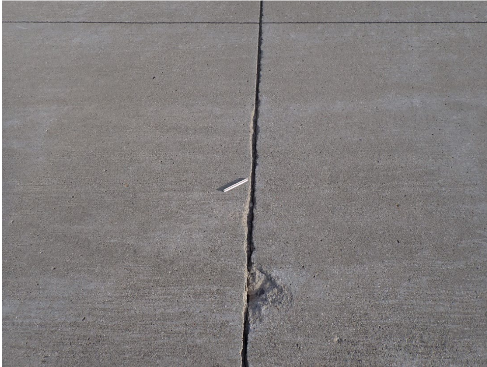
TH01NE-01. Joint Spalling (Sample Unit No. 03).
