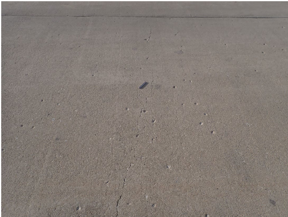
T08NE-02. LTD Cracking (Sample Unit No. 01).
