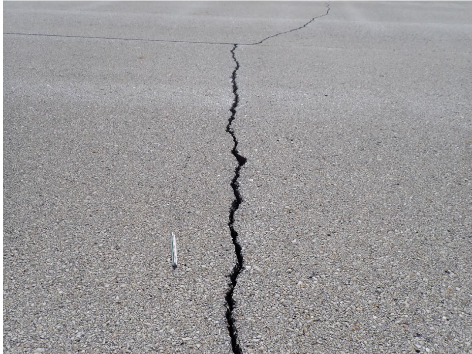
R14NE-03. L&T Cracking (Sample Unit No. 04).
