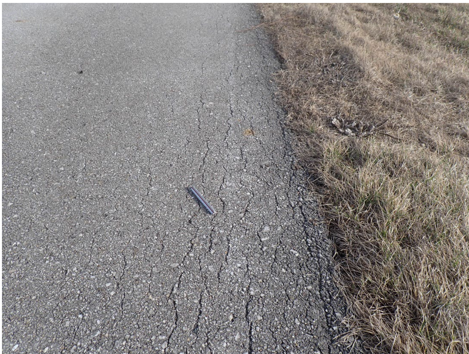
T05NE-01. Alligator Cracking (Sample Unit No. 10).
