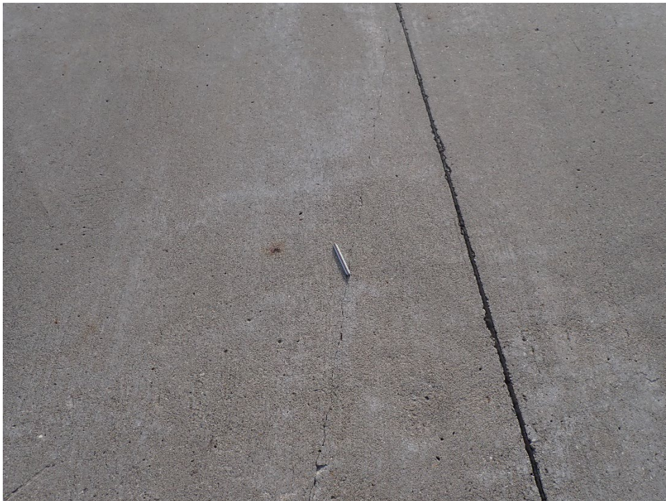
TH01NE-01. LTD Cracking (Sample Unit No. 03).
