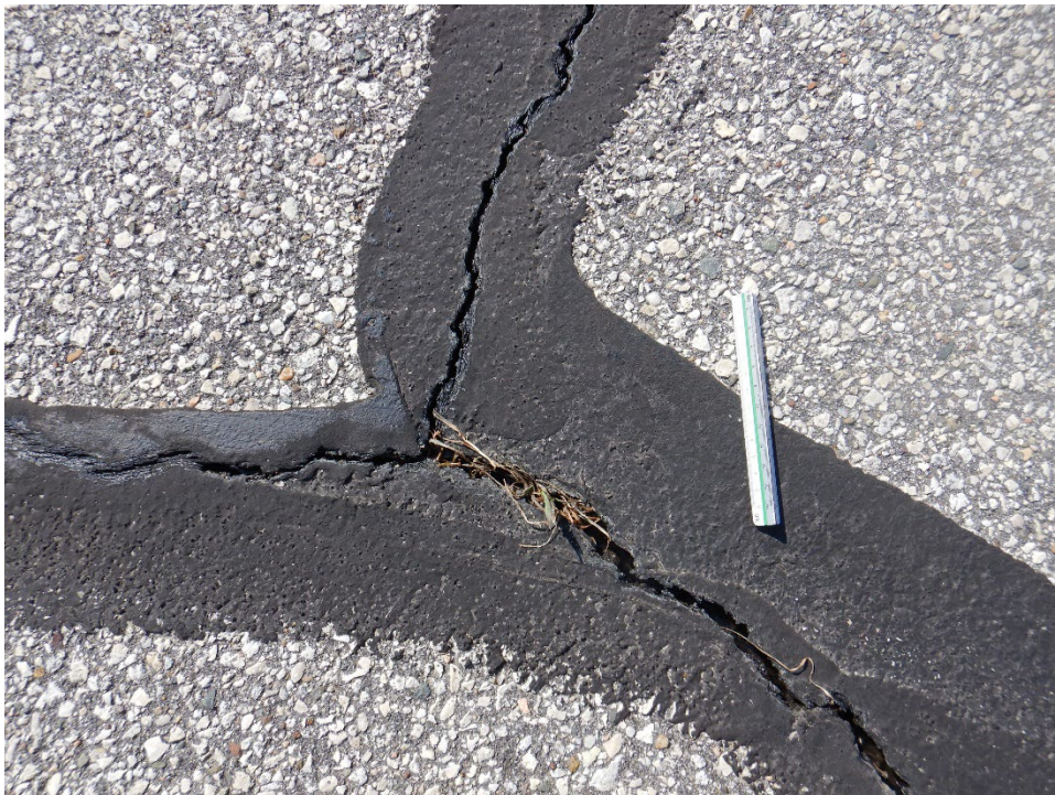
A01NH-01. L&T Cracking (Sample Unit No. 03).
