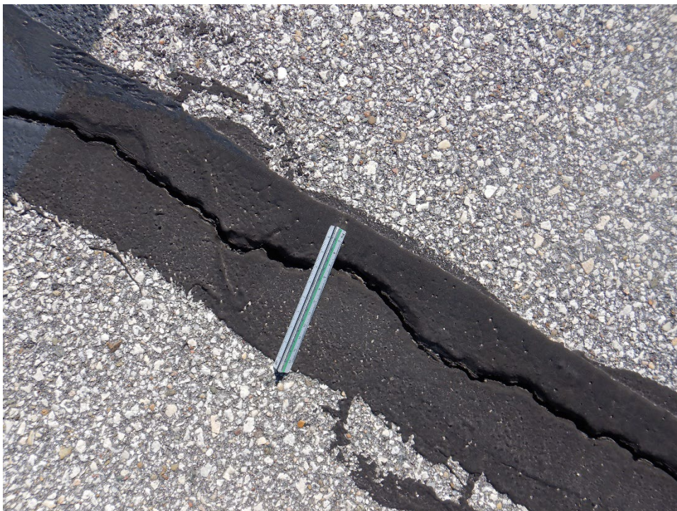
R17NH-01. L&T Cracking (Sample Unit No. 06).
