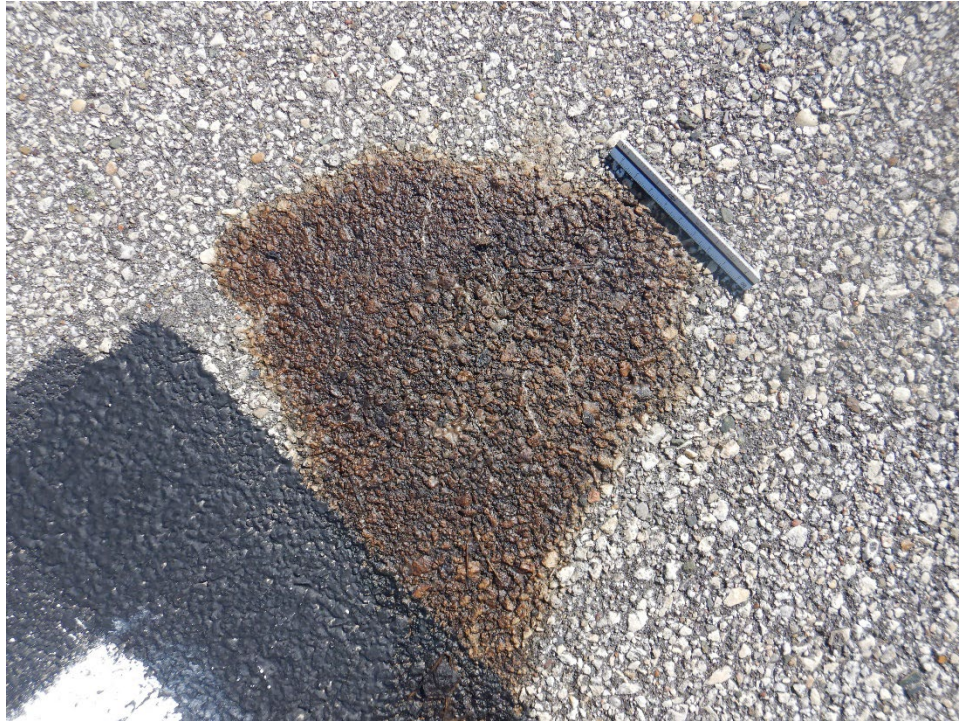
R17NH-01. Oil-Fuel Damage (Sample Unit No. 11).
