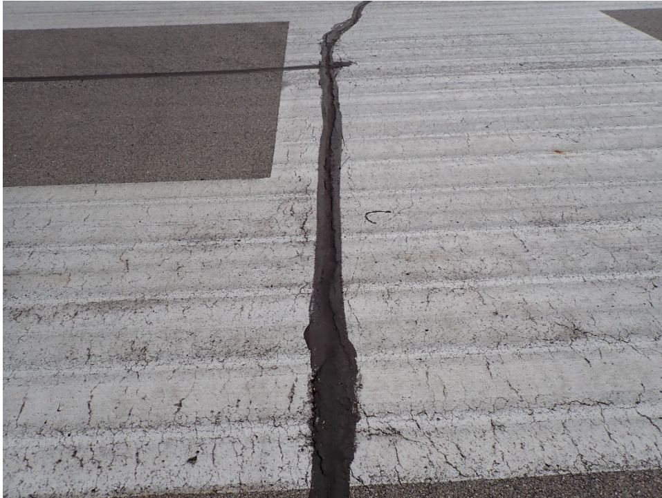
R09MD-03. L&T Cracking (Sample Unit No. 02).
