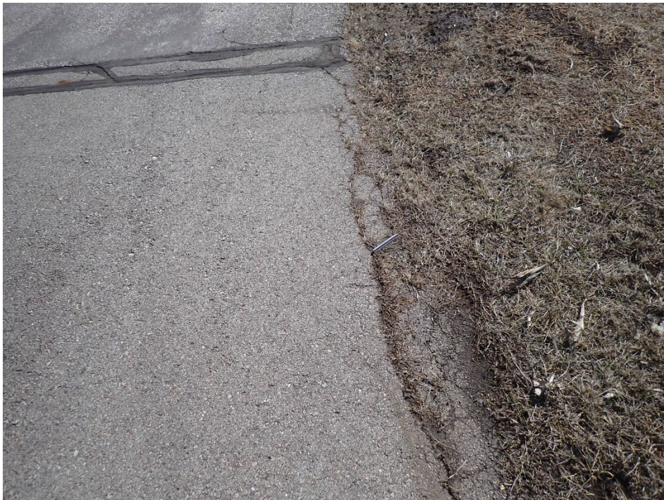
T01MD-02. Alligator Cracking (Sample Unit No. 01).
