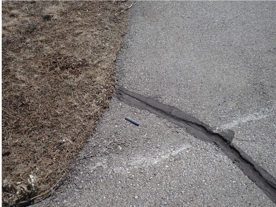
T01MD-02. L&T Cracking (Sample Unit No. 01).
