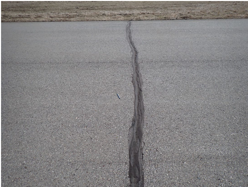
R09MD-01. L&T Cracking (Sample Unit No. 18).
