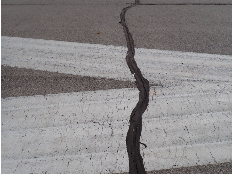
R09MD-02. L&T Cracking (Sample Unit No. 01).
