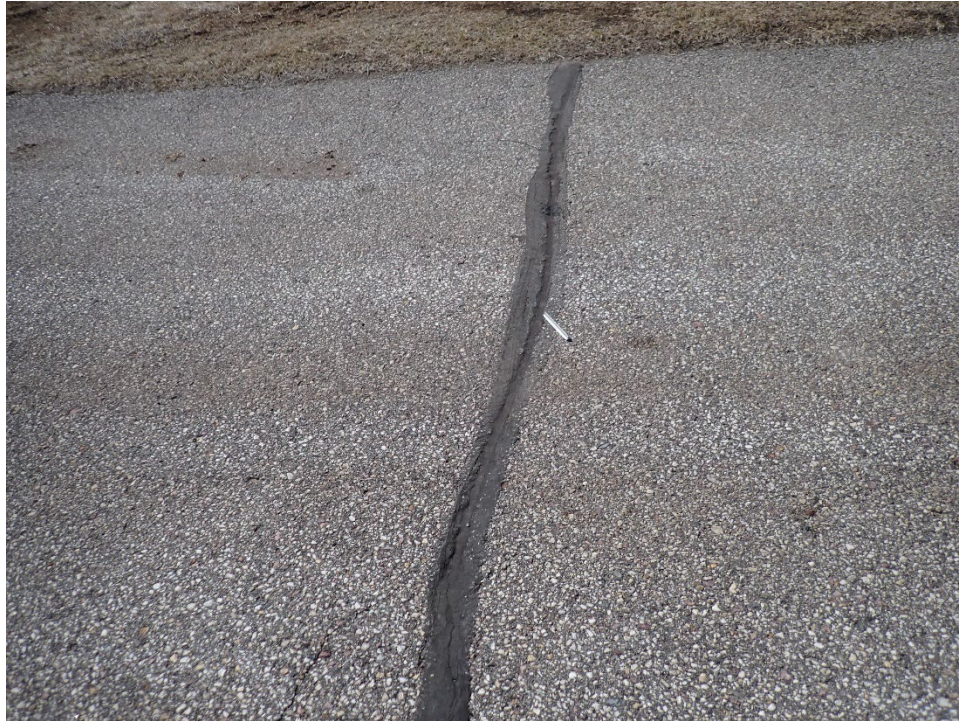
T01MD-01. L&T Cracking (Sample Unit No. 02).
