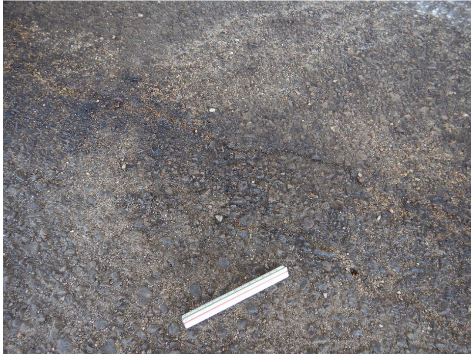
A01MC-60. Oil-Fuel Damage (Sample Unit No. 03) (2).
