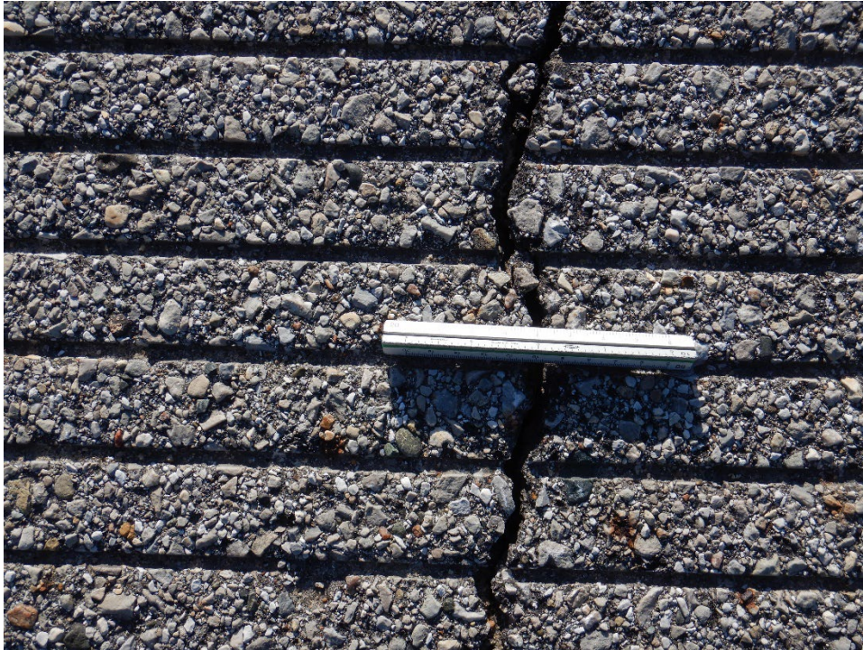
R12MC-40. L&T Cracking (Sample Unit No. 01).
