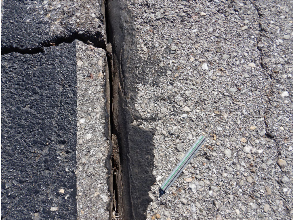
TAMC-20. L&T Cracking (Sample Unit No. 01) (2).
