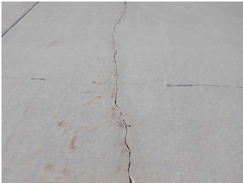
A01MC-40. LTD Cracking (Sample Unit No. 02).
