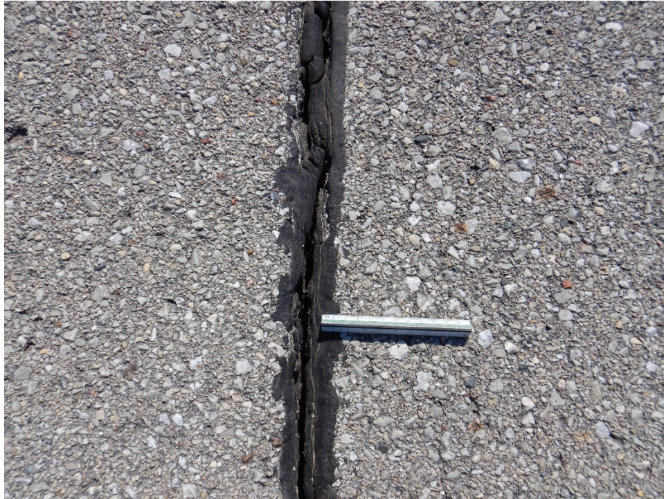
TBMC-30. L&T Cracking (Sample Unit No. 04).
