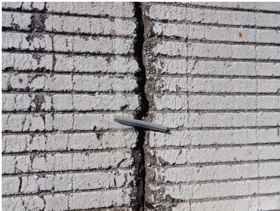
R18MC-40. L&T Cracking (Sample Unit No. 10) (2).
