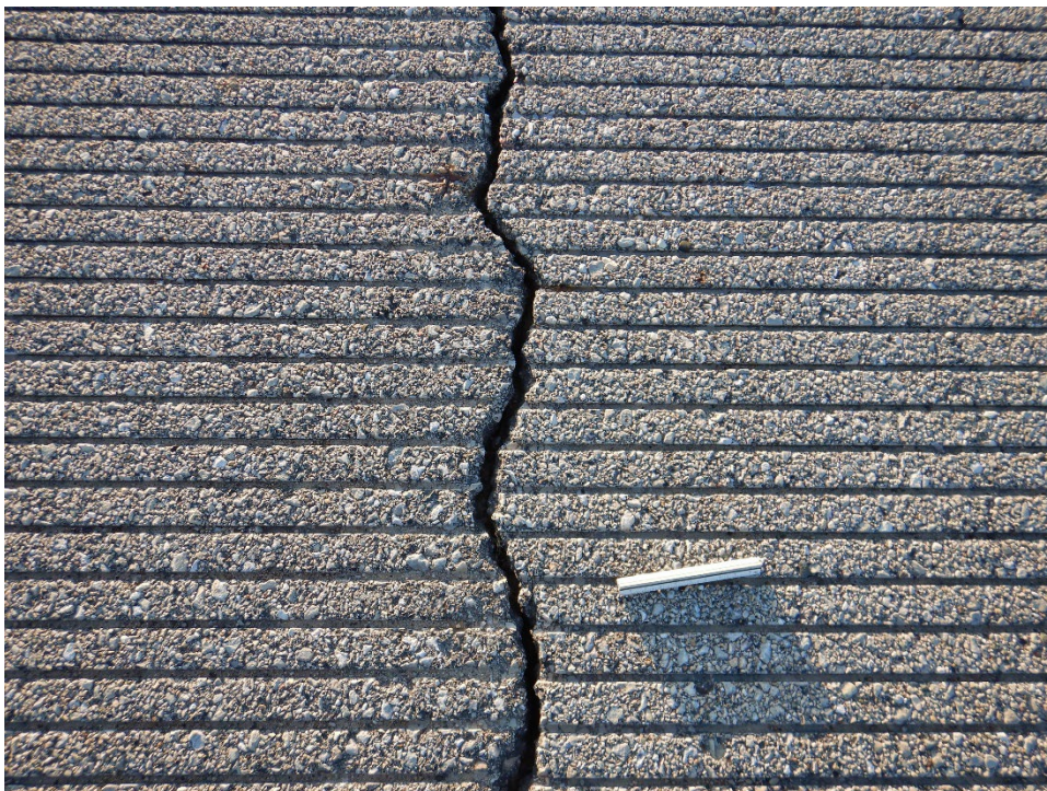
R12MC-20. L&T Cracking (Sample Unit No. 32).
