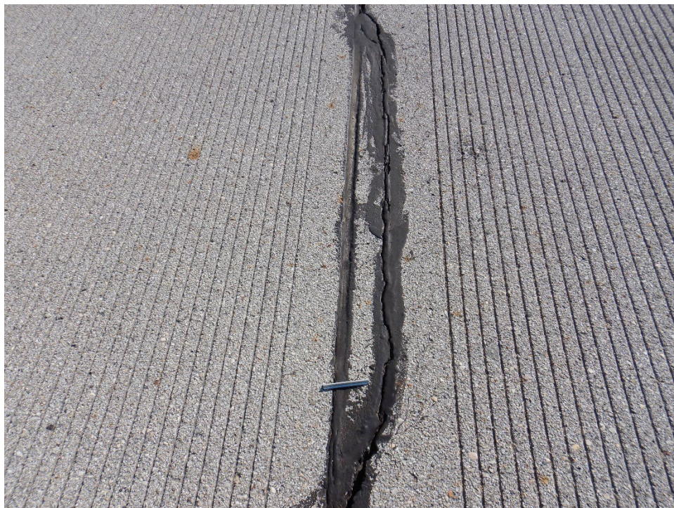
R18MC-40. L&T Cracking (Sample Unit No. 08).
