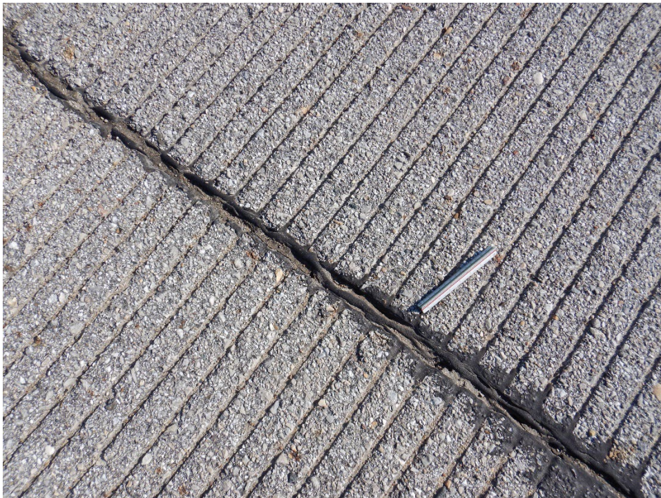
R18MC-20. L&T Cracking (Sample Unit No. 093).
