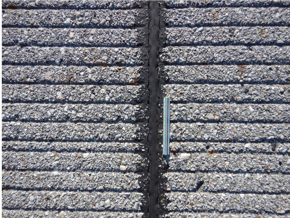
R12MC-30. L&T Cracking (Sample Unit No. 01).
