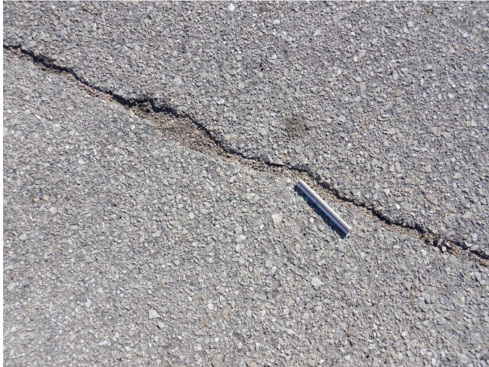
A01MC-60. L&T Cracking (Sample Unit No. 04).
