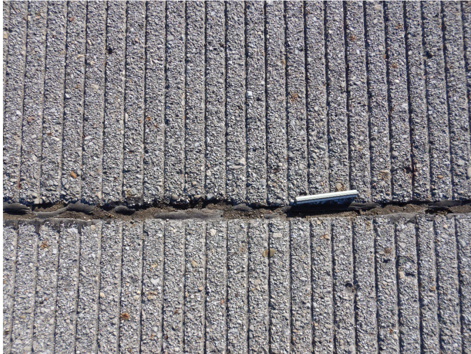
R18MC-60. L&T Cracking (Sample Unit No. 18).
