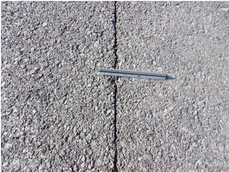
A01MC-35. L&T Cracking (Sample Unit No. 09).
