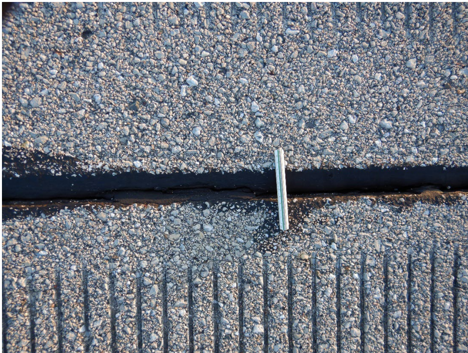
R12MC-10. L&T Cracking (Sample Unit No. 43).
