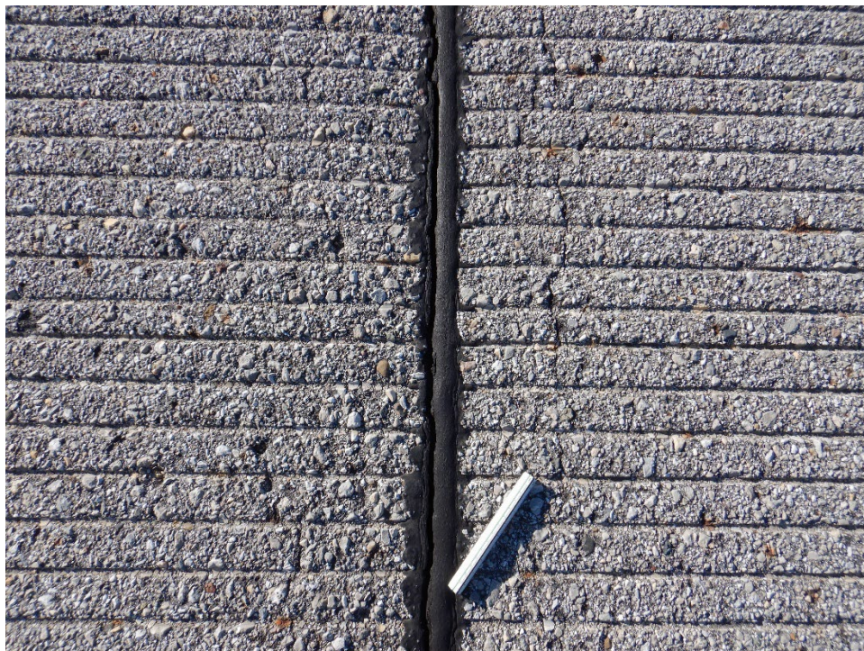
R18MC-50. L&T Cracking (Sample Unit No. 07).
