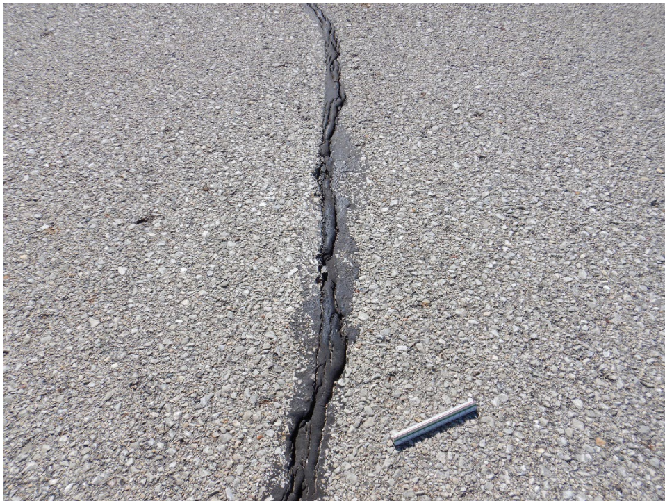
A01MC-50. L&T Cracking (Sample Unit No. 01).
