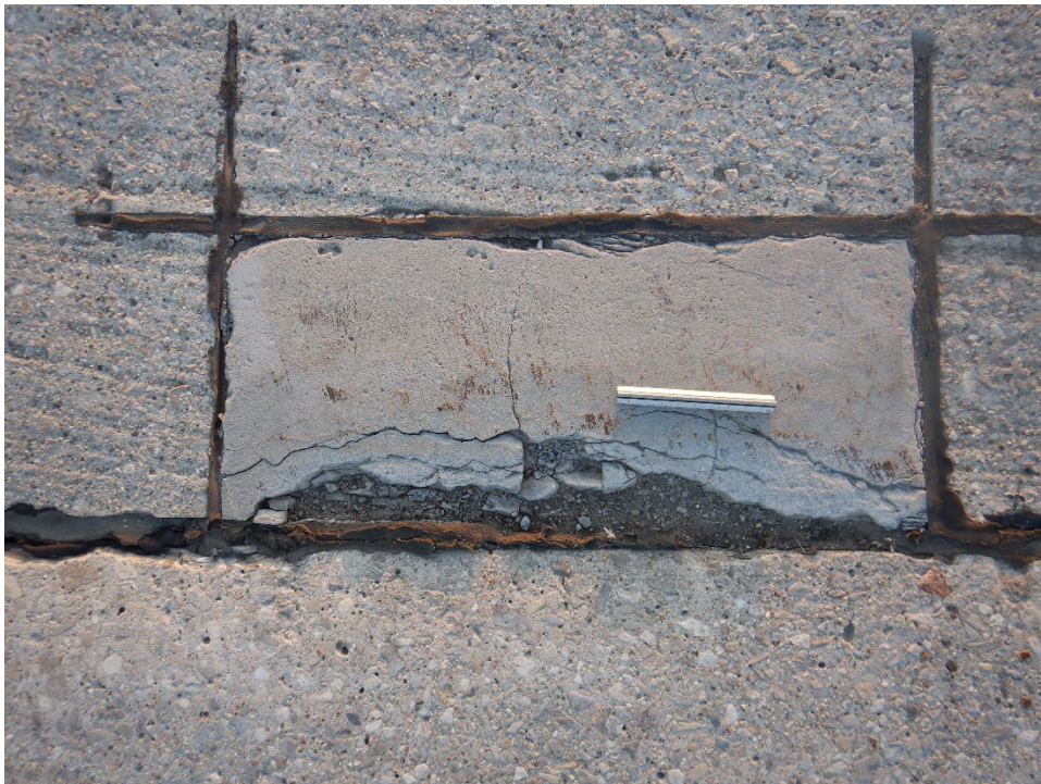
A01MC-20. Small Patching (Sample Unit No. 02).
