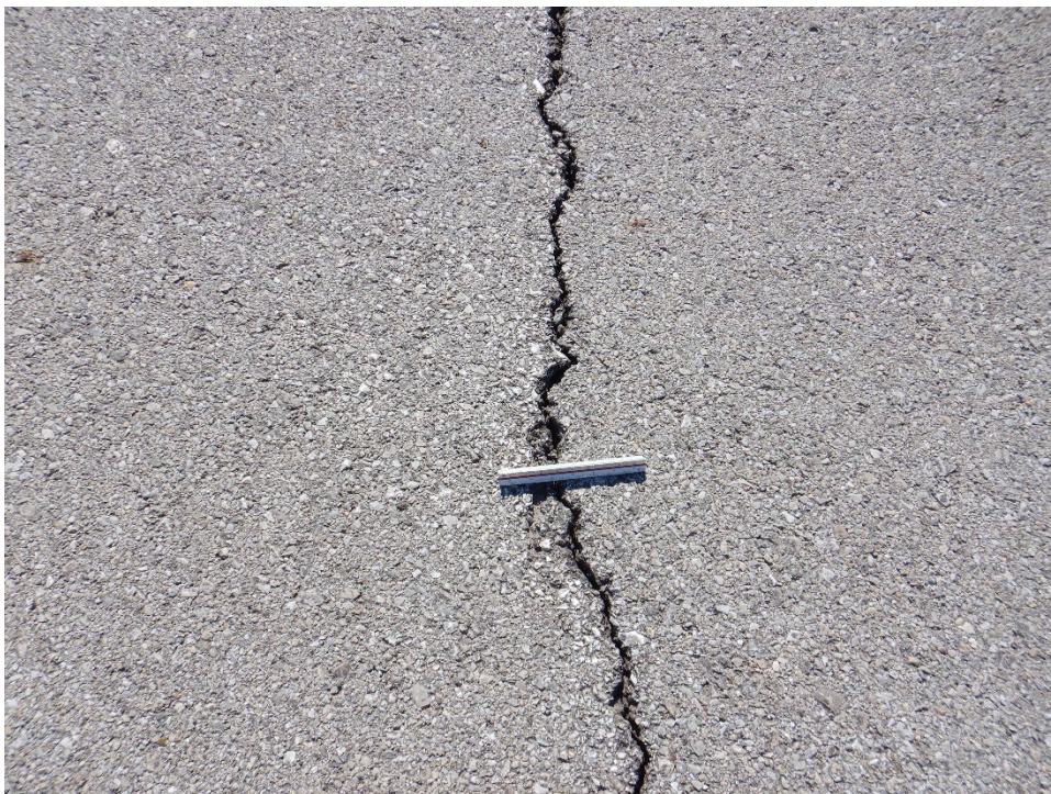
TAMC-30. L&T Cracking (Sample Unit No. 04).
