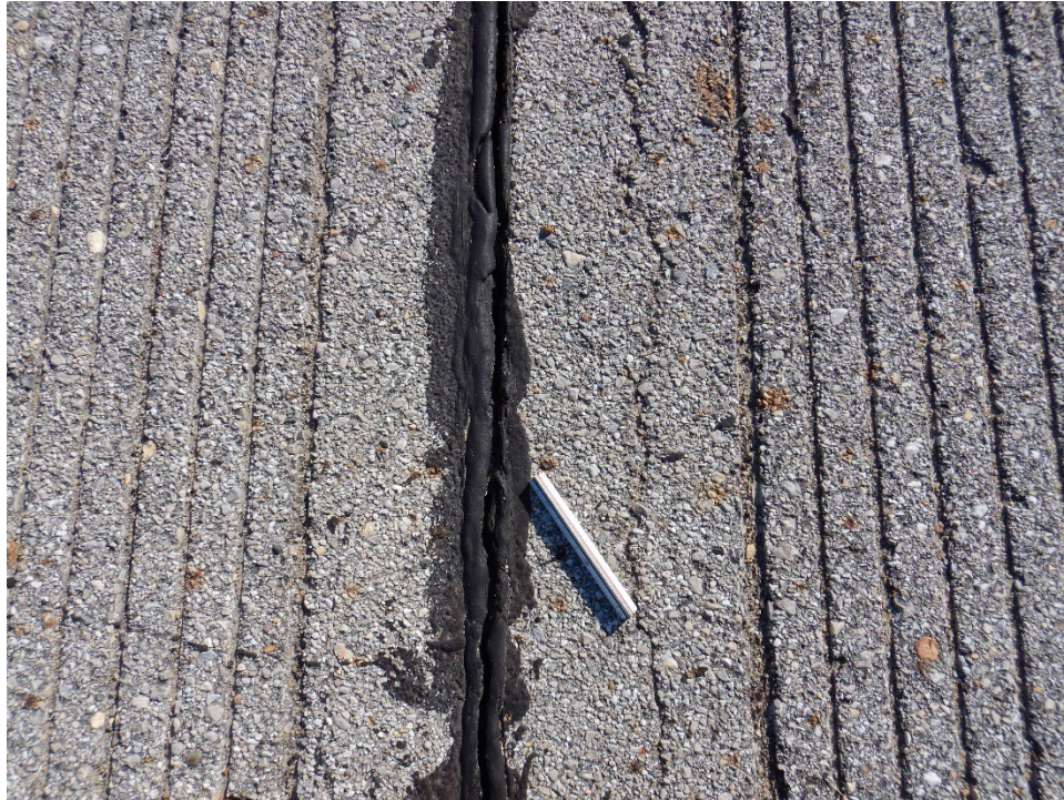
R18MC-40. L&T Cracking (Sample Unit No. 10) (1).
