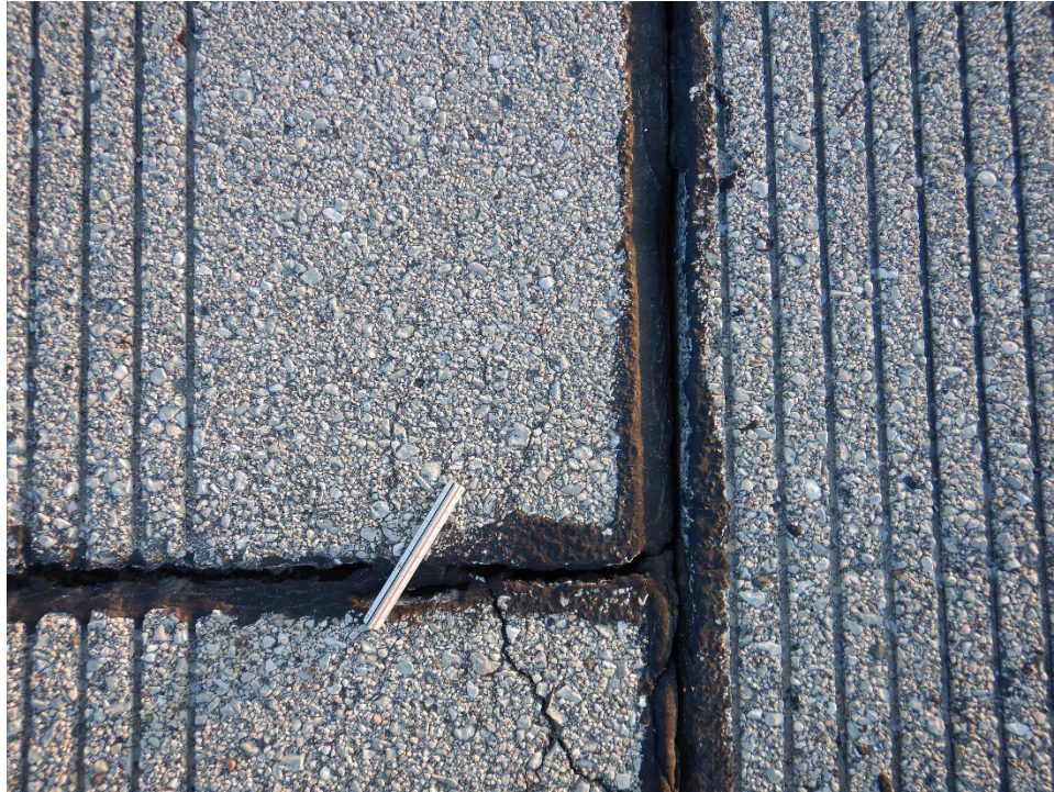
R12MC-20. L&T Cracking (Sample Unit No. 42).
