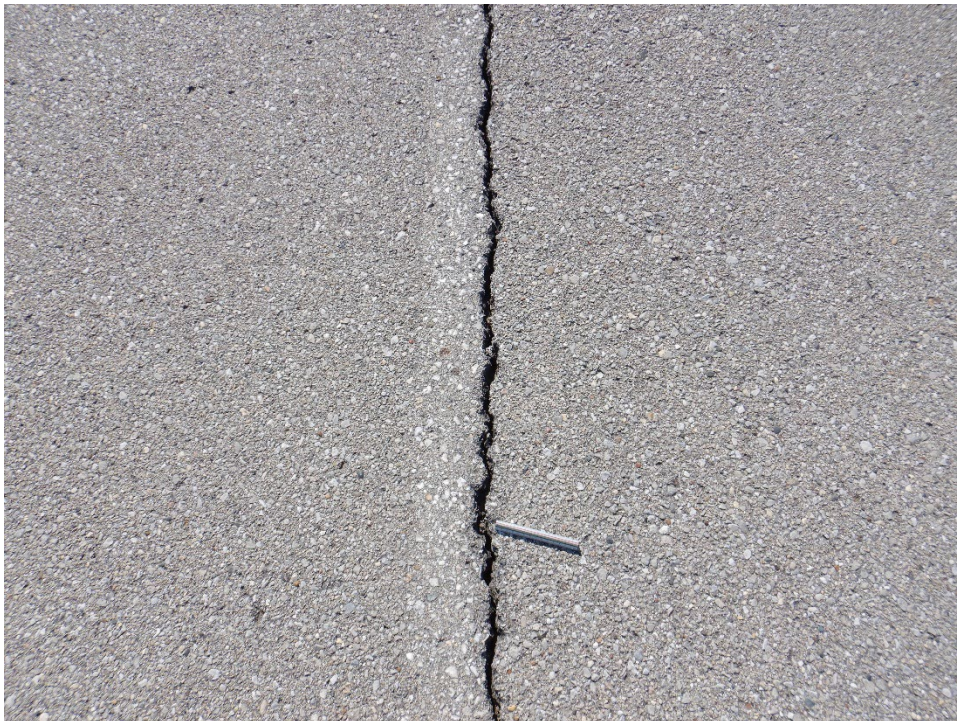
TCMC-10. L&T Cracking (Sample Unit No. 14).
