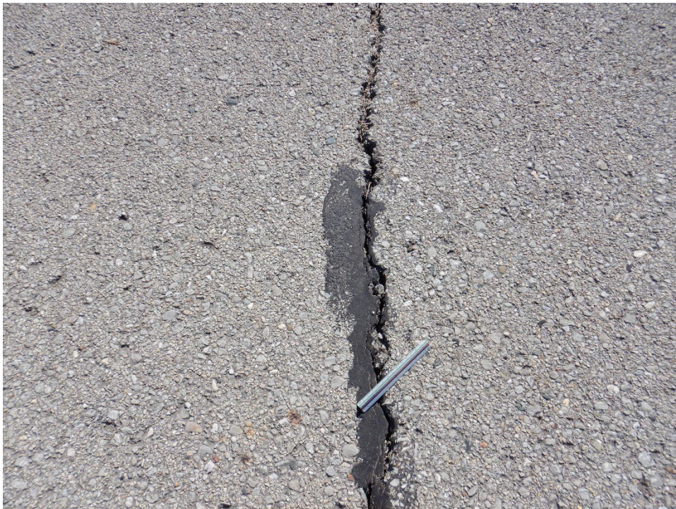
TBMC-35. L&T Cracking (Sample Unit No. 01).
