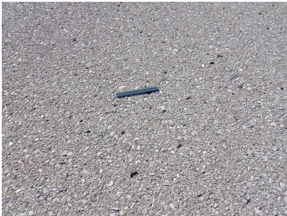
TBMC-30. Raveling (Sample Unit No. 04).
