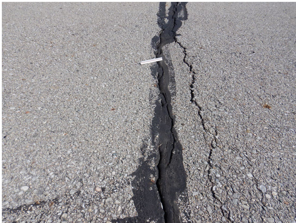
TAMC-10. L&T Cracking (Sample Unit No. 48).
