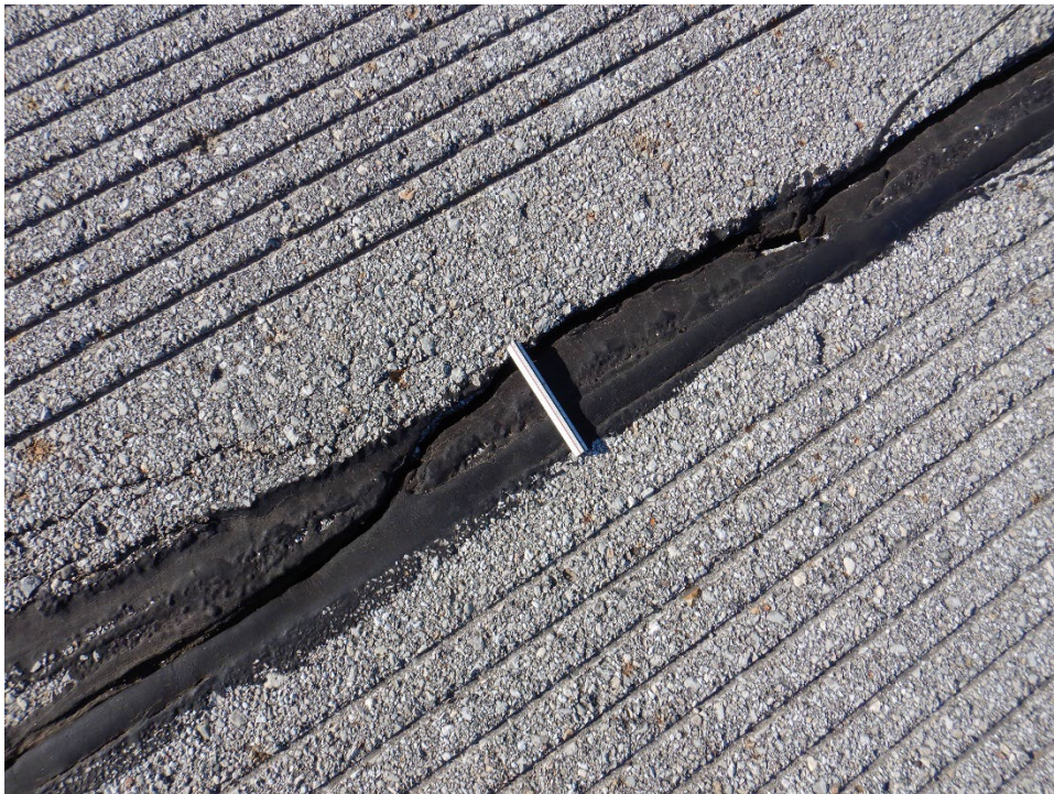
R18MC-60. L&T Cracking (Sample Unit No. 06).
