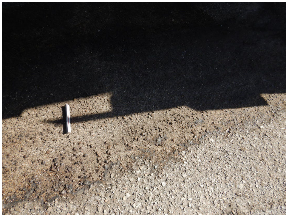
A01MC-60. Oil-Fuel Damage (Sample Unit No. 03) (1).
