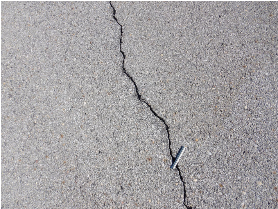
TAMC-20. L&T Cracking (Sample Unit No. 01) (1).
