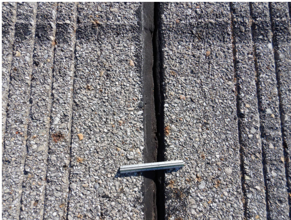
R18MC-30. L&T Cracking (Sample Unit No. 05).
