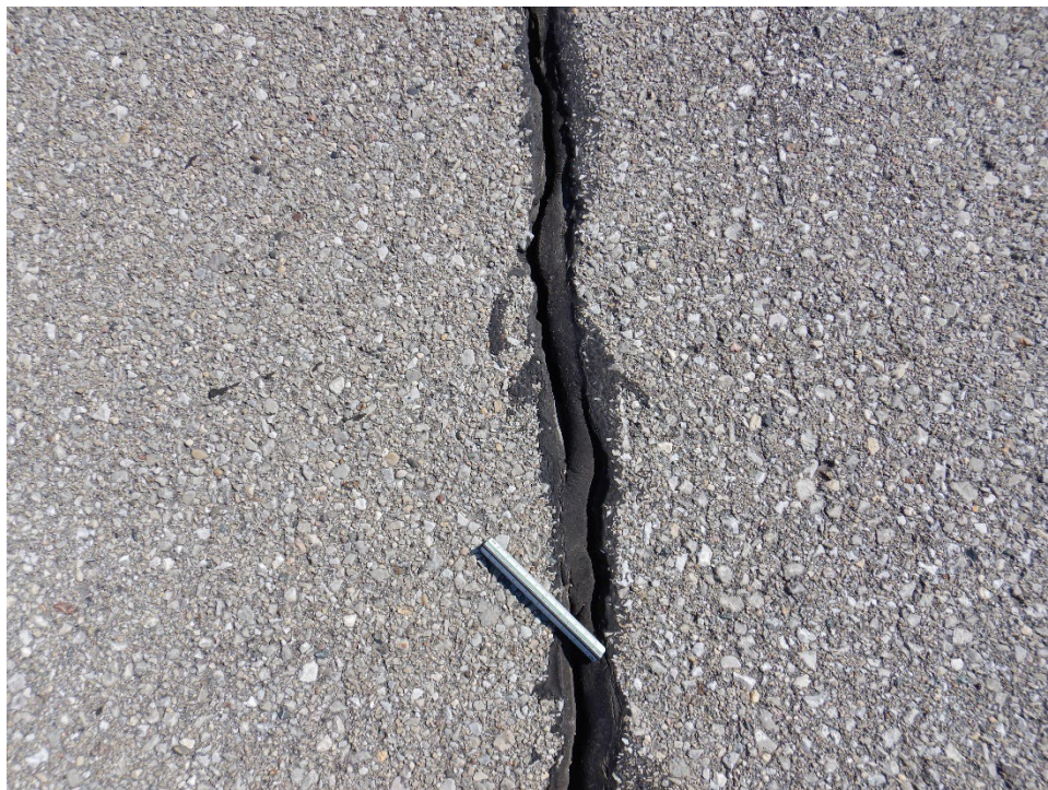
TCMC-10. L&T Cracking (Sample Unit No. 39).
