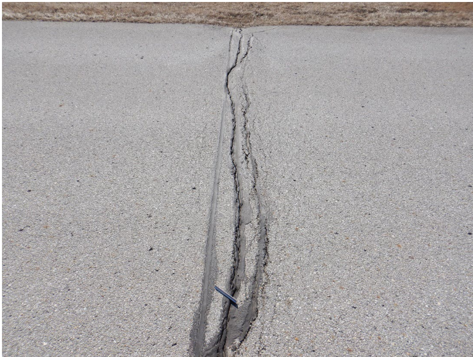
TBMC-25. L&T Cracking (Sample Unit No. 02).
