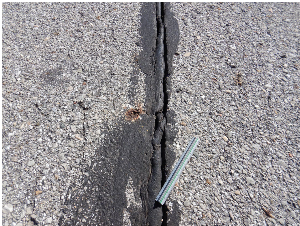
TCMC-20. L&T Cracking (Sample Unit No. 01) (1).
