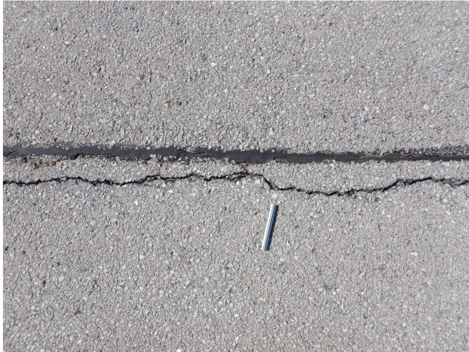
TBMC-10. L&T Cracking (Sample Unit No. 02).
