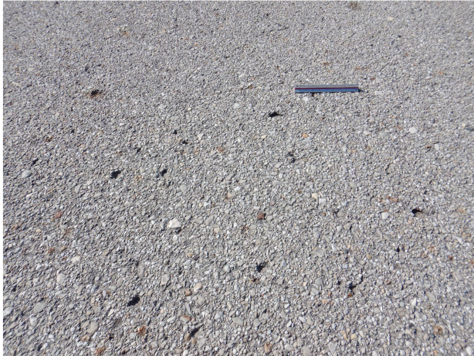
TBMC-25. Raveling (Sample Unit No. 01).
