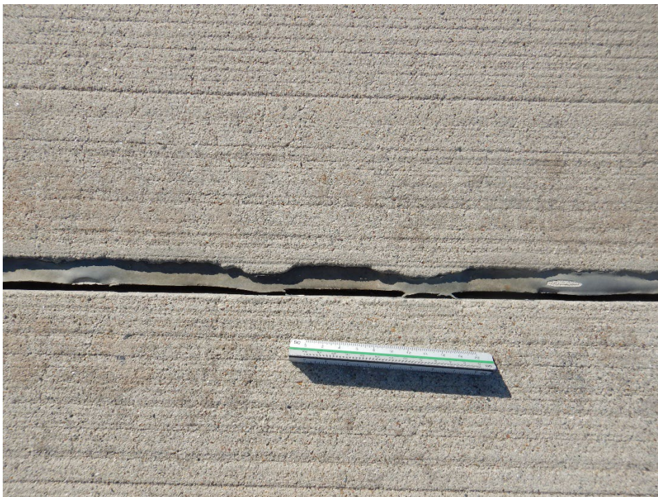
A01MC-10. Joint Seal Damage (Sample Unit No. 01).
