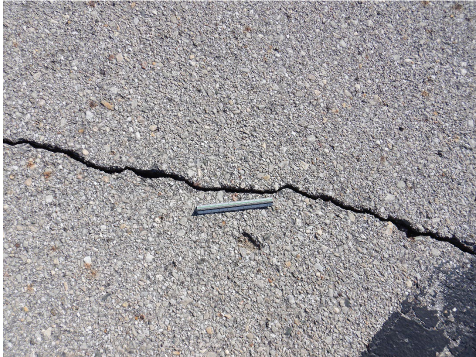
TCMC-20. L&T Cracking (Sample Unit No. 01) (2).
