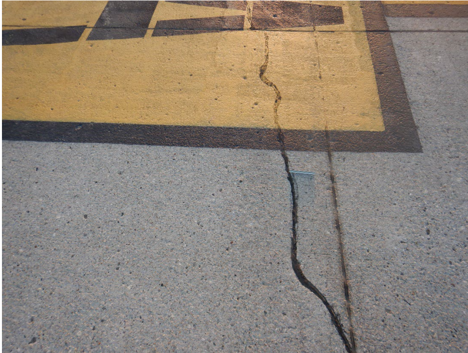
A01MC-20. LTD Cracking (Sample Unit No. 02) (2).
