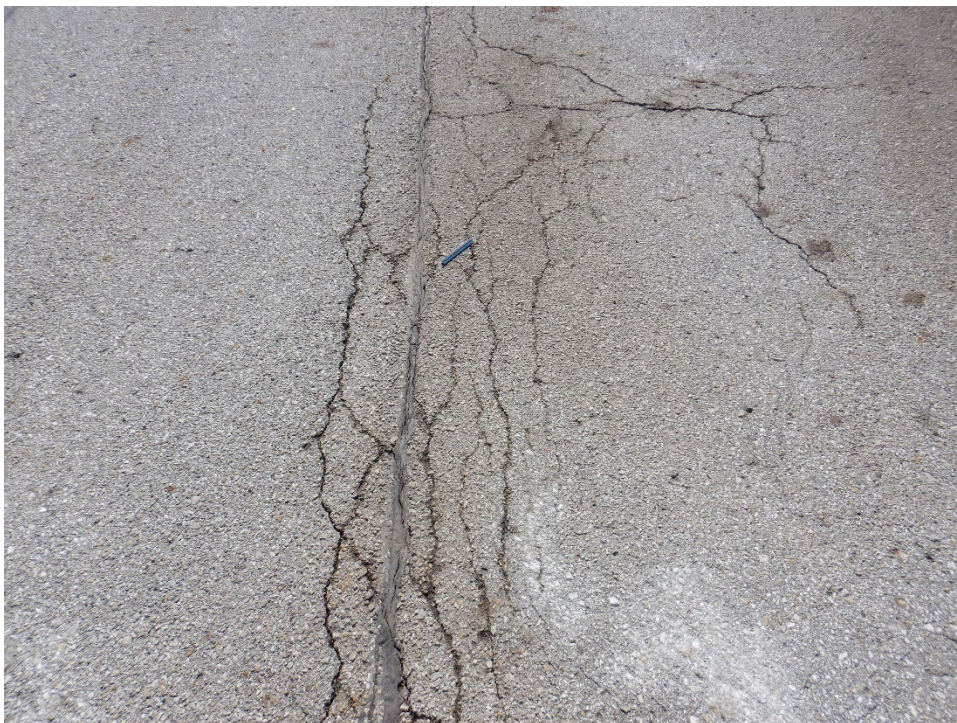
TH01MC-20. Alligator Cracking (Sample Unit No. 01).
