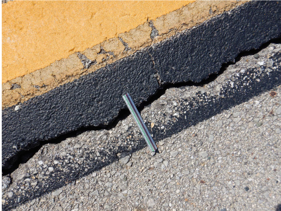
TAMC-10. L&T Cracking (Sample Unit No. 40).
