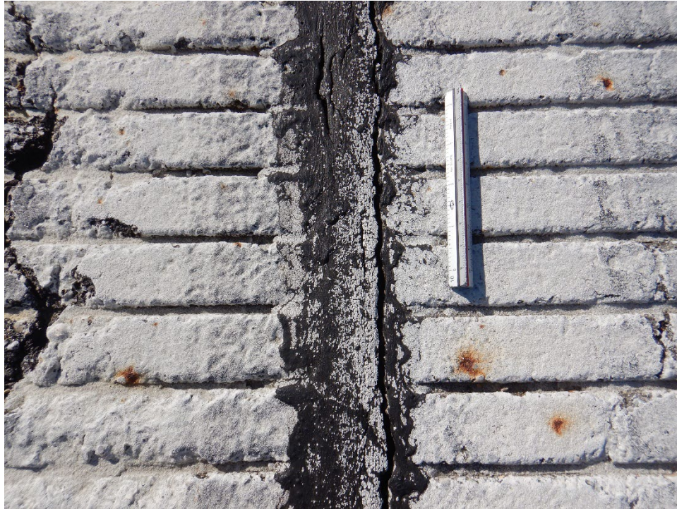
R18MC-10. L&T Cracking (Sample Unit No. 42).
