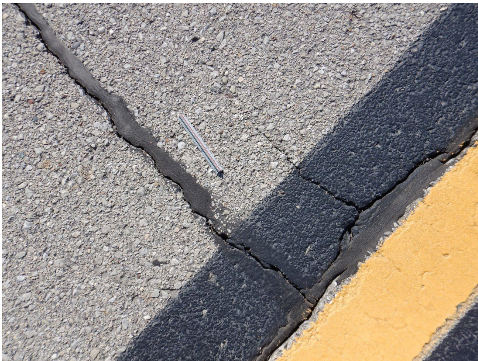
TBMC-15. L&T Cracking (Sample Unit No. 01).
