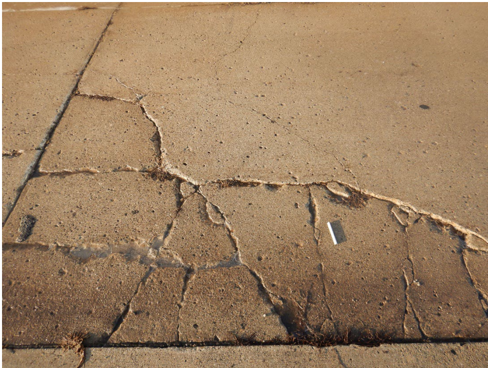
TH01MC-30. Shattered Slab (Sample Unit No. 18) (2).
