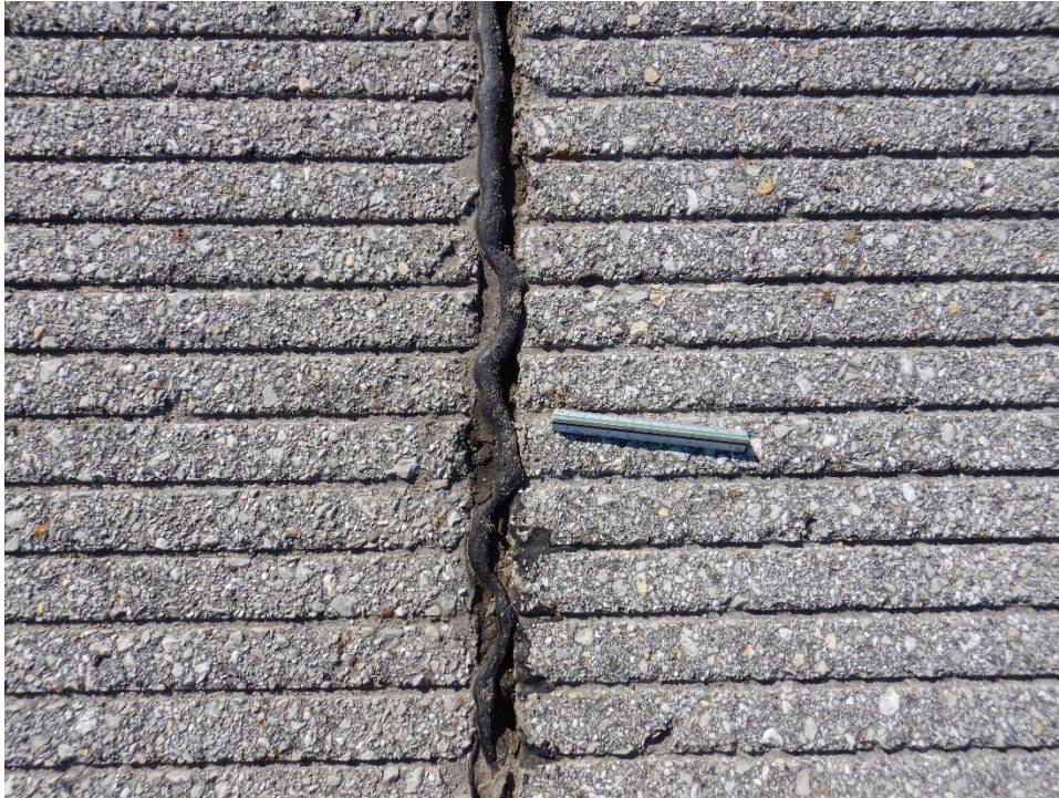
R18MC-20. L&T Cracking (Sample Unit No. 021).
