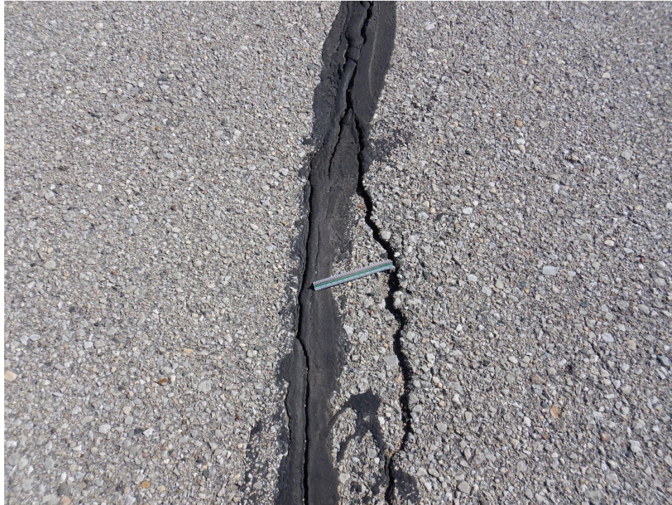
TCMC-10. L&T Cracking (Sample Unit No. 24).
