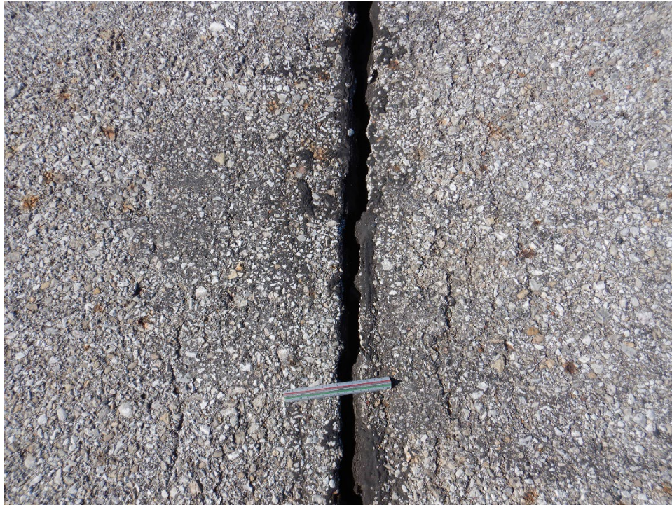
TH01MC-20. L&T Cracking (Sample Unit No. 01).
