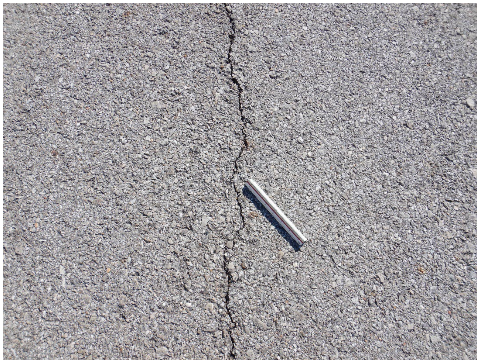
TH01MC-35. L&T Cracking (Sample Unit No. 02).
