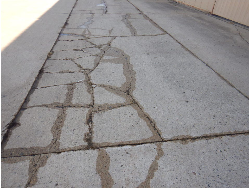
TH01MC-30. Shattered Slab (Sample Unit No. 18) (1).
