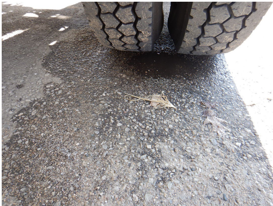
A01MC-60. Rutting (Sample Unit No. 04).
