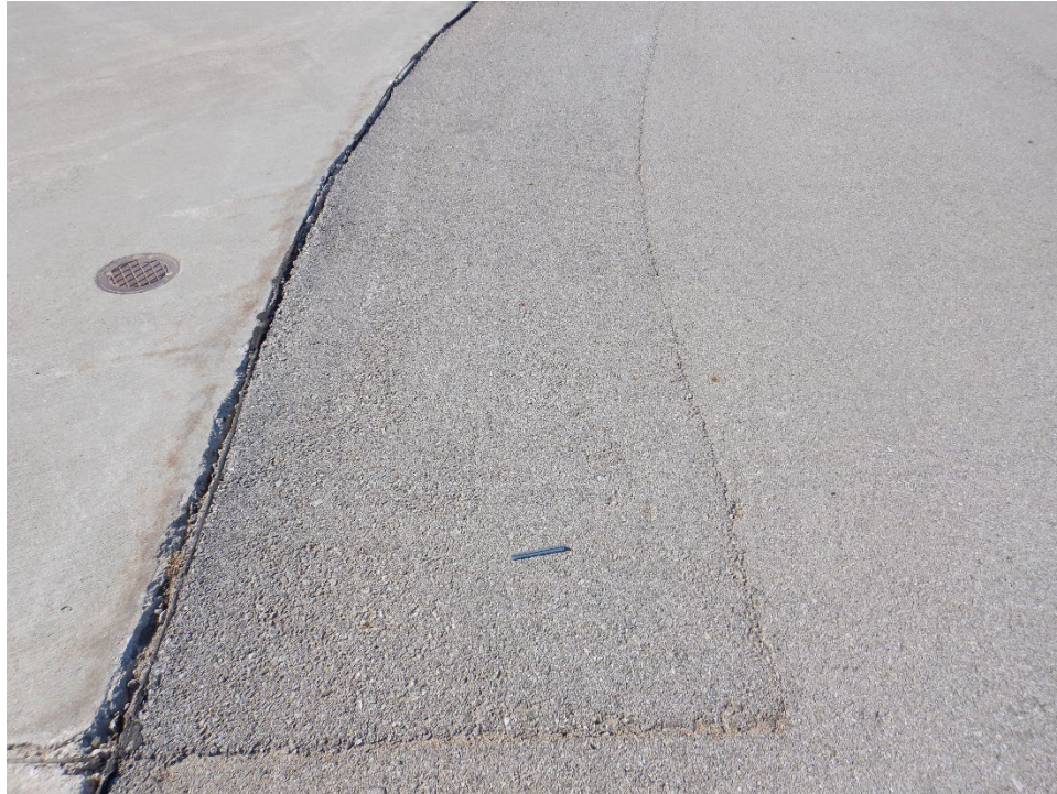
A01MC-35. Patching (Additional Sample Unit No. 13).
