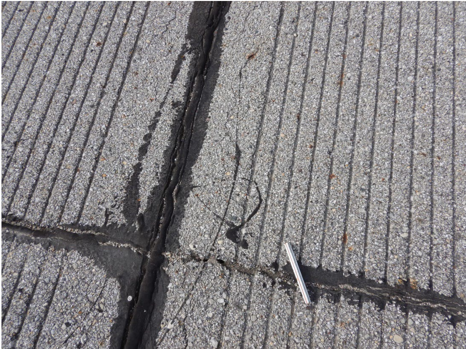
R18MC-40. L&T Cracking (Sample Unit No. 02).
