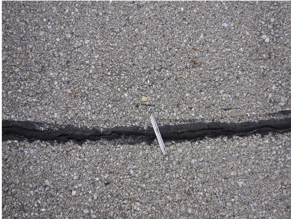
TBMC-20. L&T Cracking (Sample Unit No. 15).
