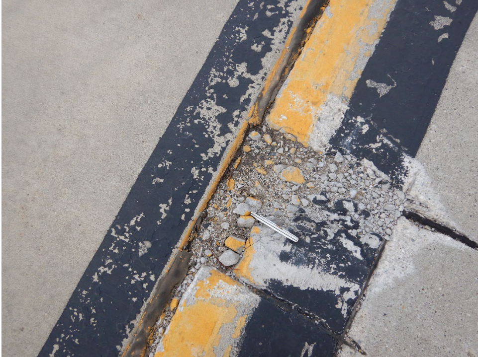
A01MC-10. Small Patching (Sample Unit No. 08).
