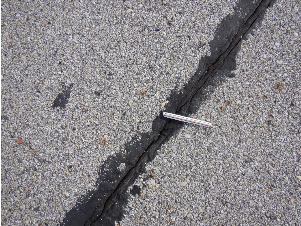
TCMC-20. L&T Cracking (Sample Unit No. 02).
