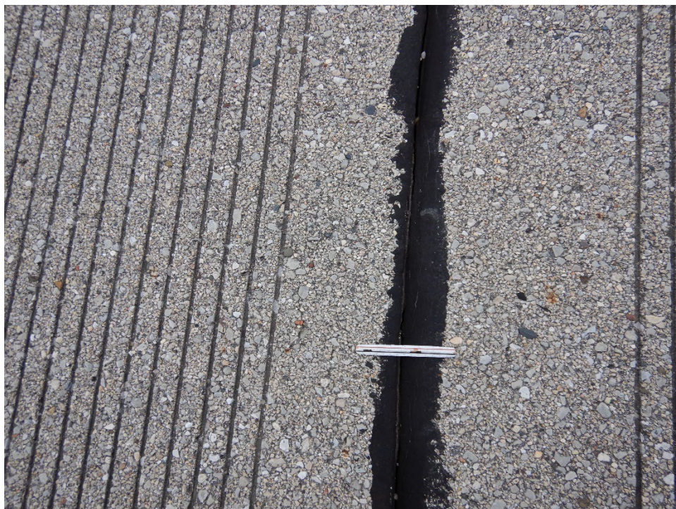
R12MC-10. L&T Cracking (Sample Unit No. 43).
