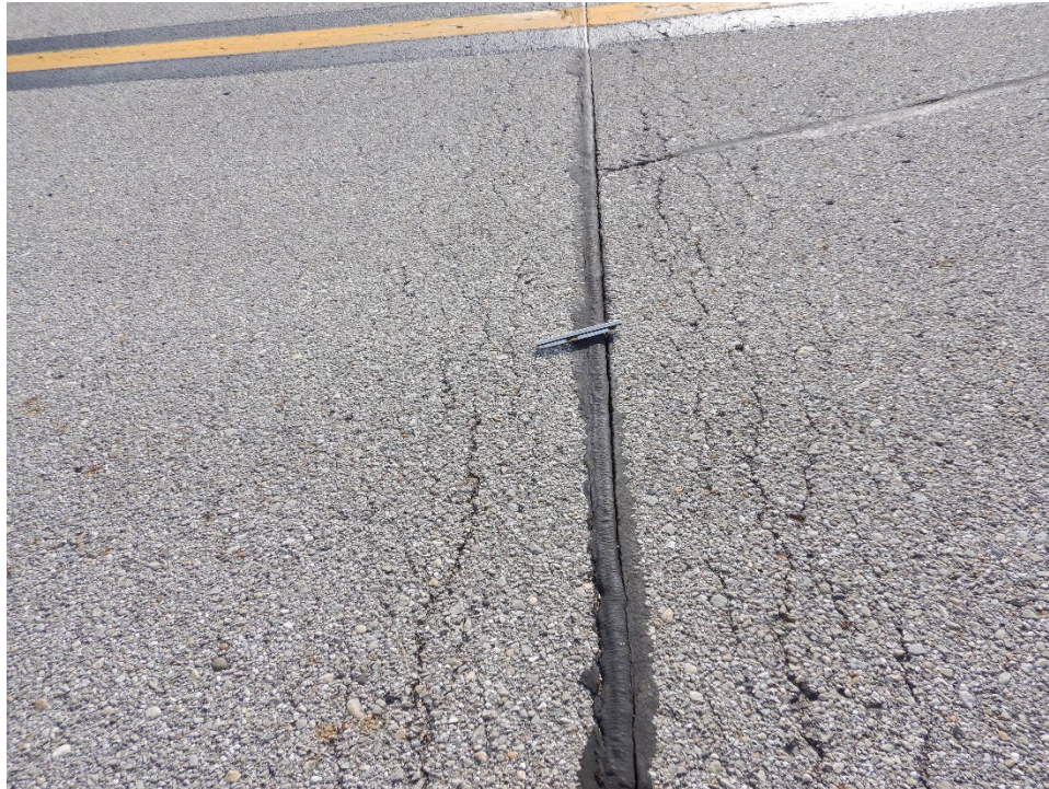
TCMC-20. L&T Cracking (Sample Unit No. 03).
