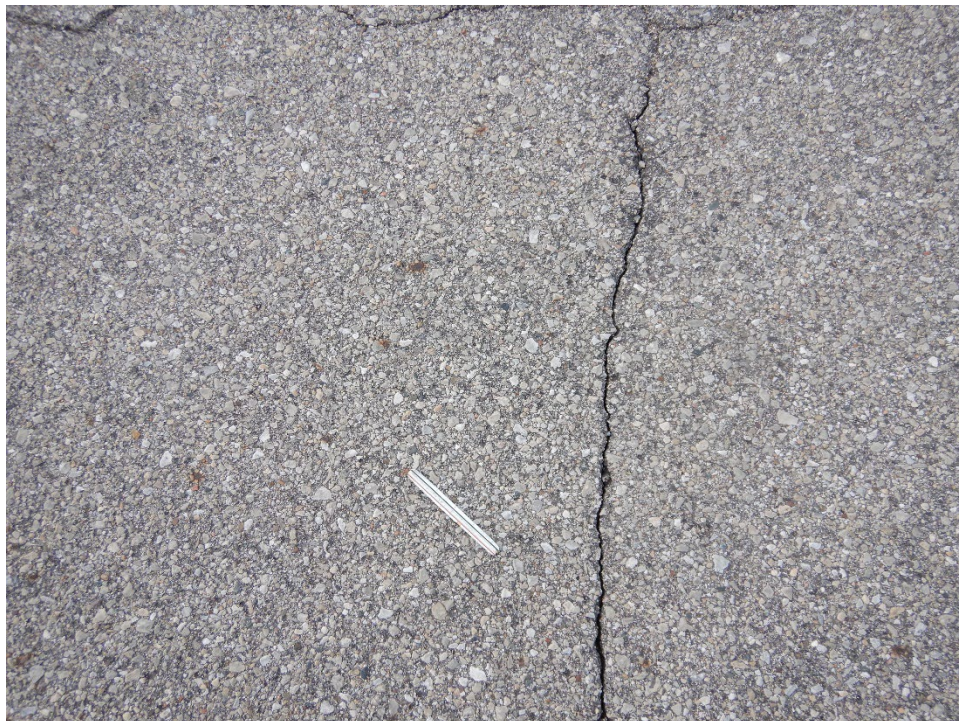
A01MC-60. L&T Cracking (Sample Unit No. 01).
