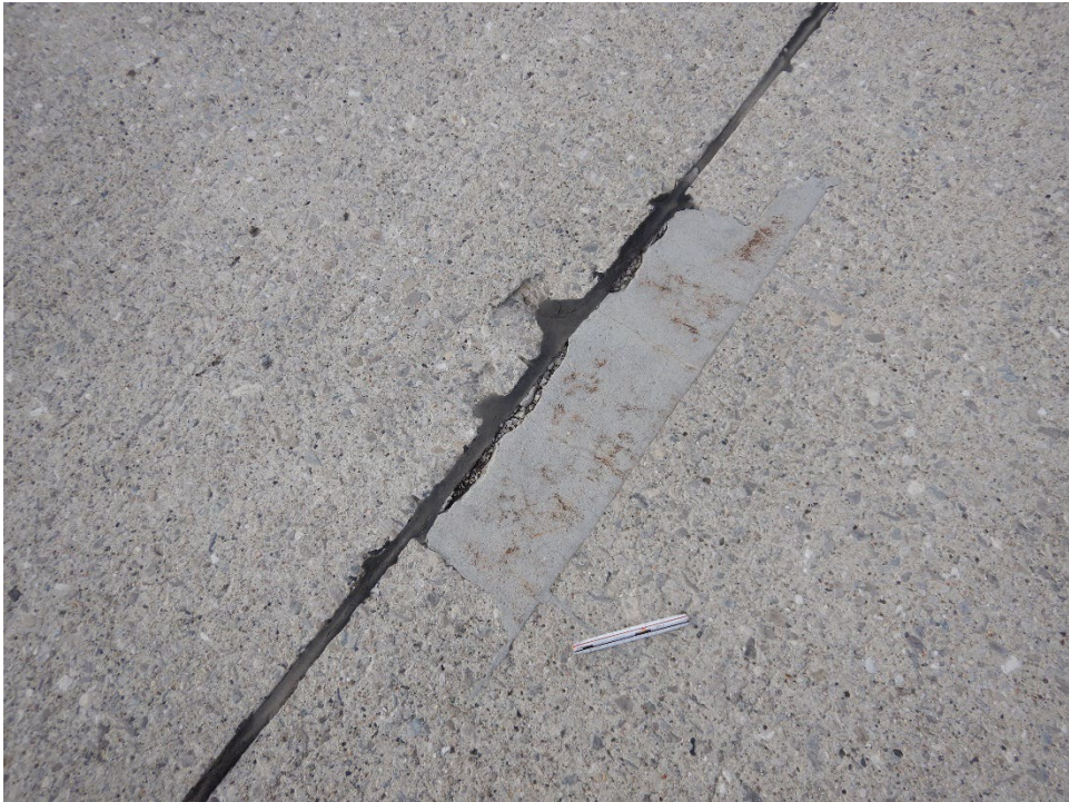
A01MC-20. Small Patching (Sample Unit No. 05).
