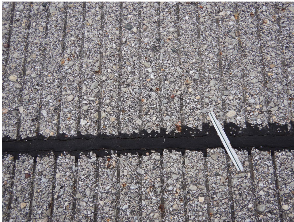
R12MC-30. L&T Cracking (Sample Unit No. 01).
