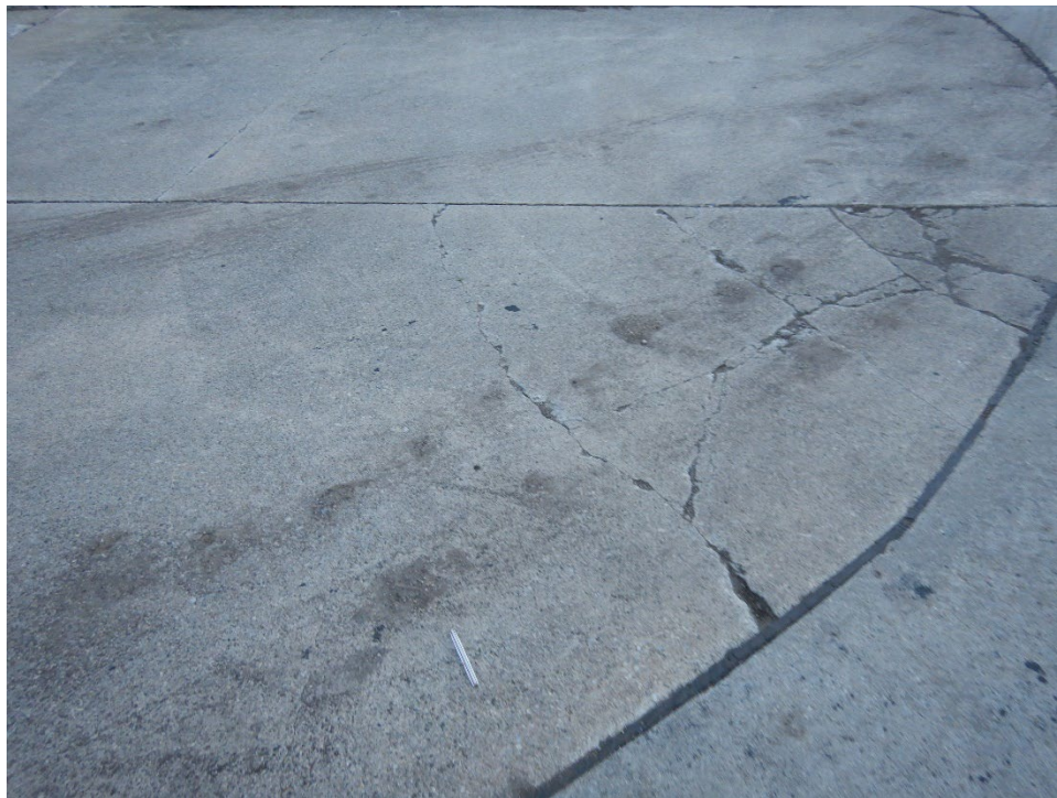
TH01MC-30. Shattered Slab (Sample Unit No. 18).
