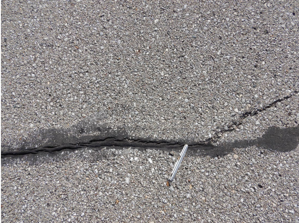
TCMC-10. L&T Cracking (Sample Unit No. 44).
