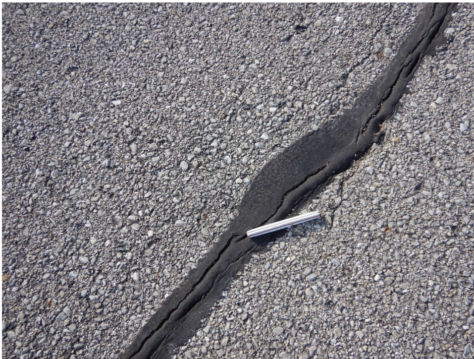
A01MC-50. L&T Cracking (Sample Unit No. 01).
