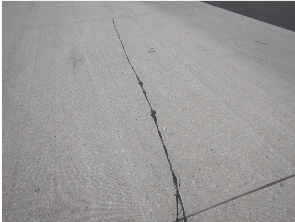
A01MC-30. LTD Cracking (Sample Unit No. 13).
