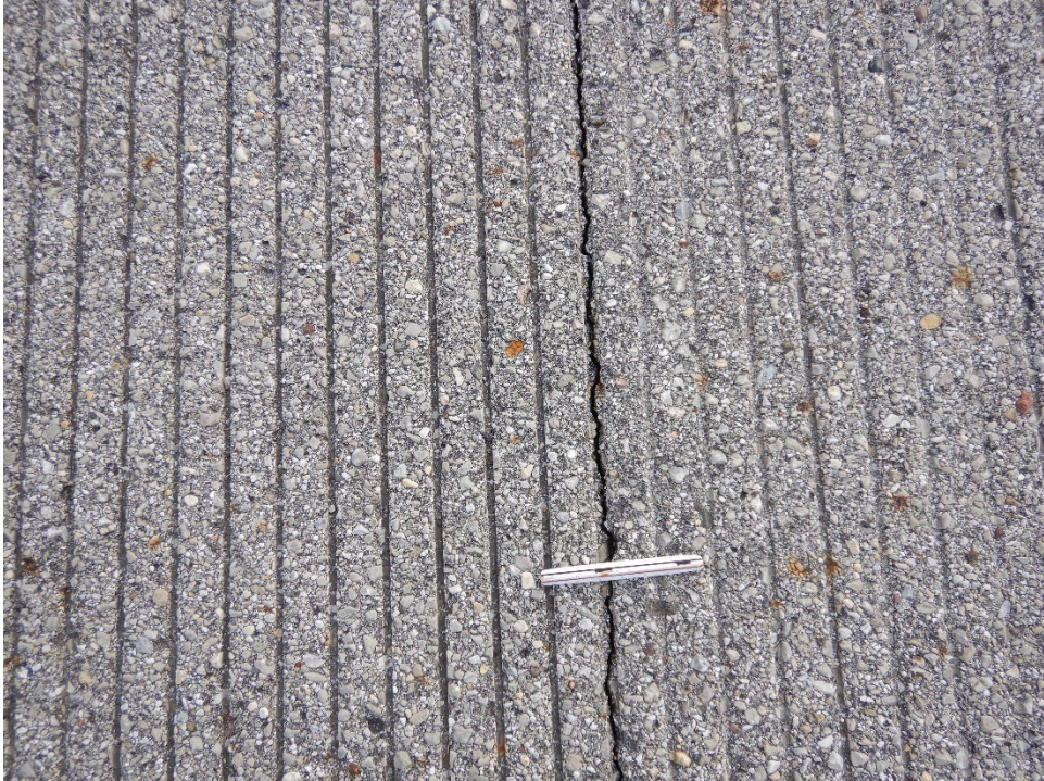
R18MC-20. L&T Cracking (Sample Unit No. 01).
