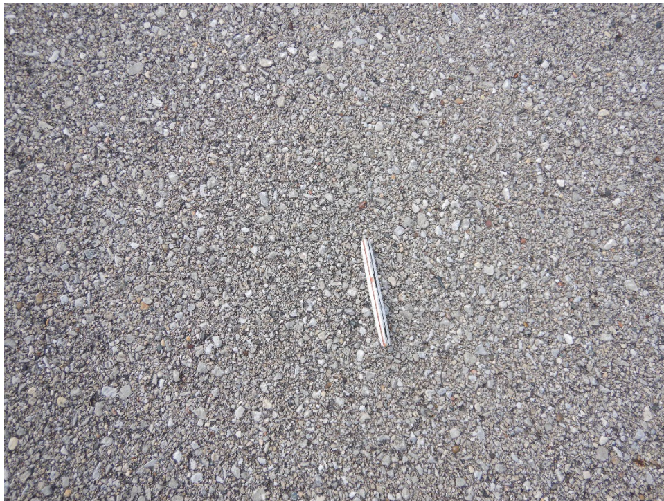
TBMC-20. Weathering (Sample Unit No. 15).
