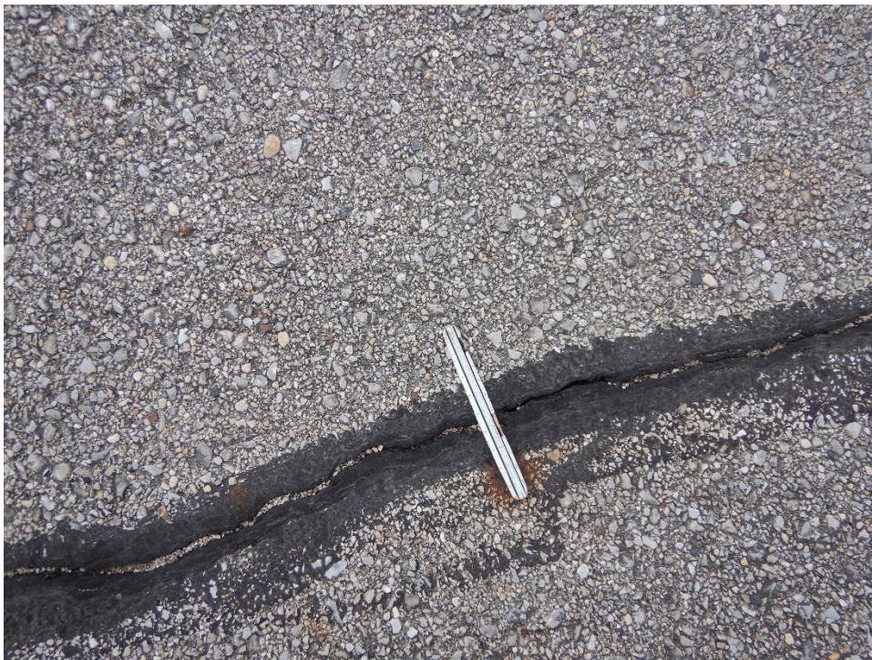
TBMC-35. L&T Cracking (Sample Unit No. 02).
