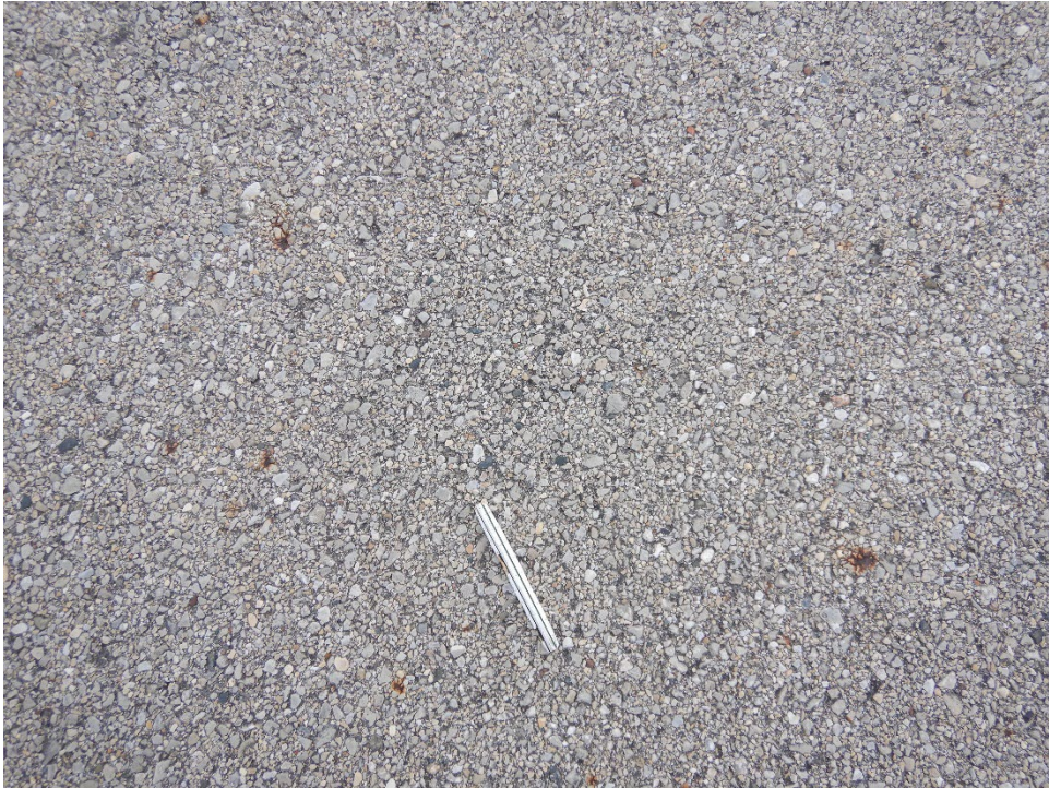
TBMC-10. Weathering (Sample Unit No. 04).
