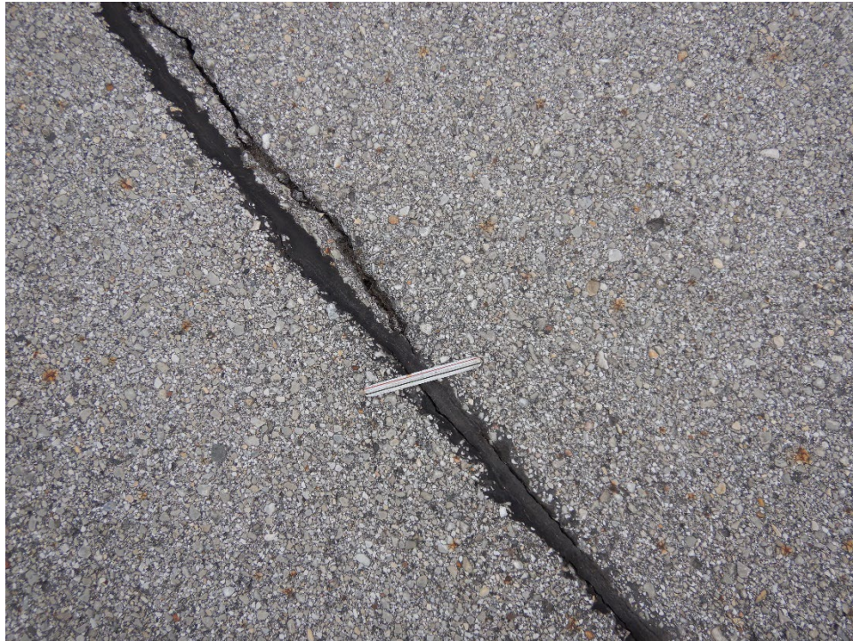
TAMC-20. L&T Cracking (Sample Unit No. 02).
