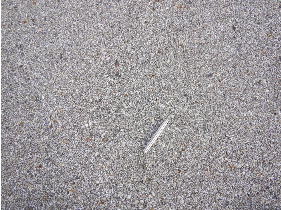
TBMC-25. Weathering (Sample Unit No. 02).
