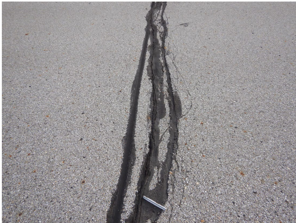
TBMC-25. L&T Cracking (Sample Unit No. 02).
