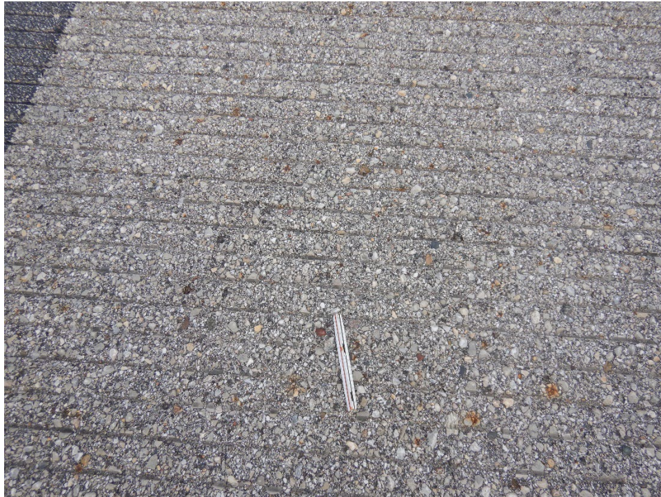
R18MC-10. Weathering (Sample Unit No. 02).
