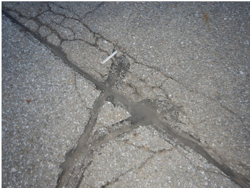
TH01MC-10. Alligator Cracking (Sample Unit No. 01).
