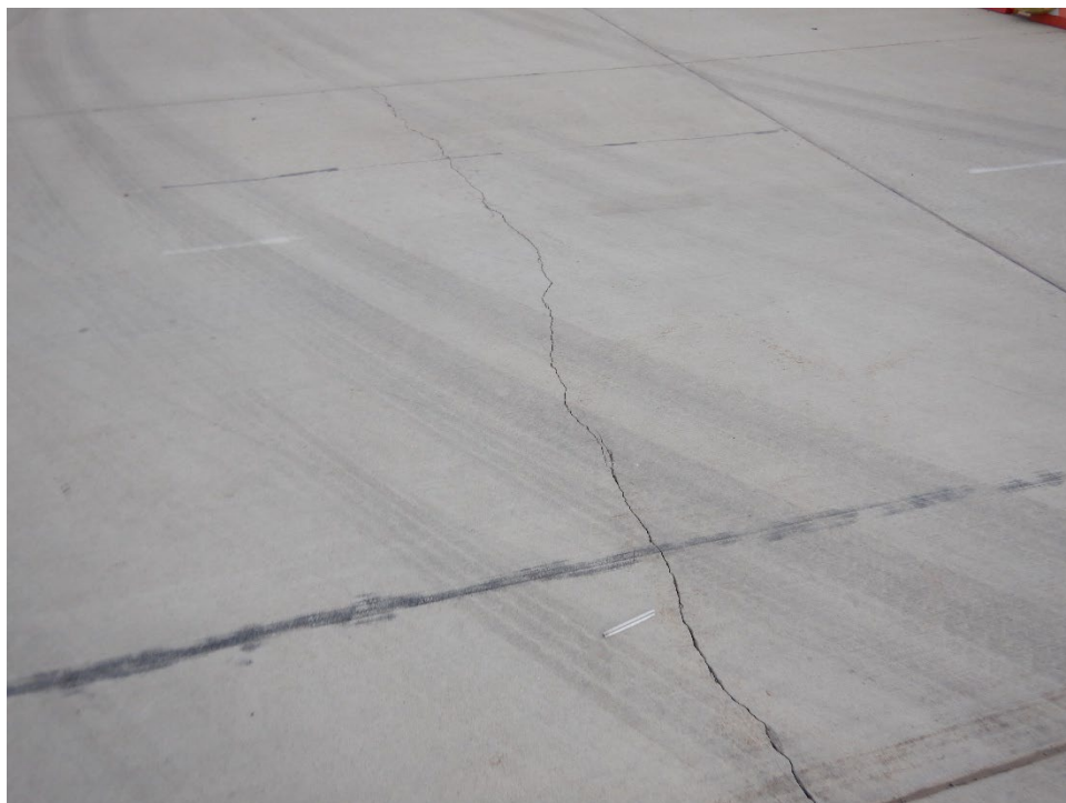
A01MC-40. LTD Cracking (Sample Unit No. 02).
