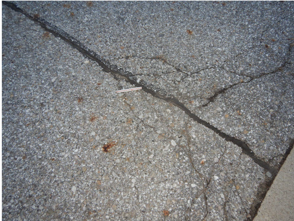
TH01MC-20. Alligator Cracking (Sample Unit No. 01).
