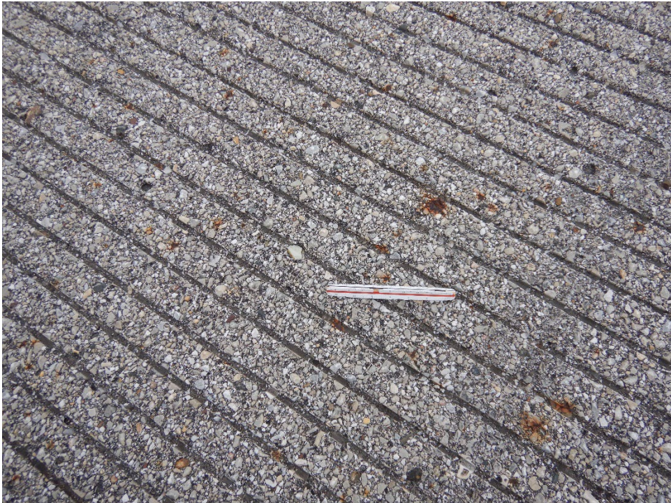
R12MC-30. Weathering (Sample Unit No. 01).
