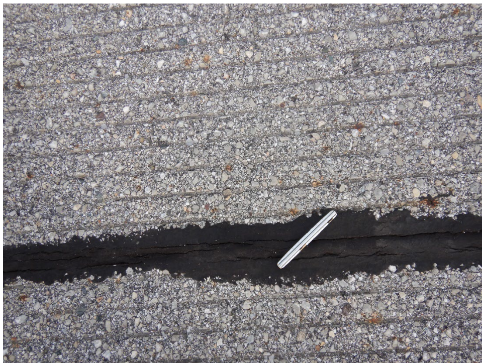
R18MC-10. L&T Cracking (Sample Unit No. 02).
