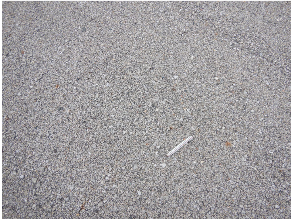
TBMC-15. Weathering (Sample Unit No. 02).
