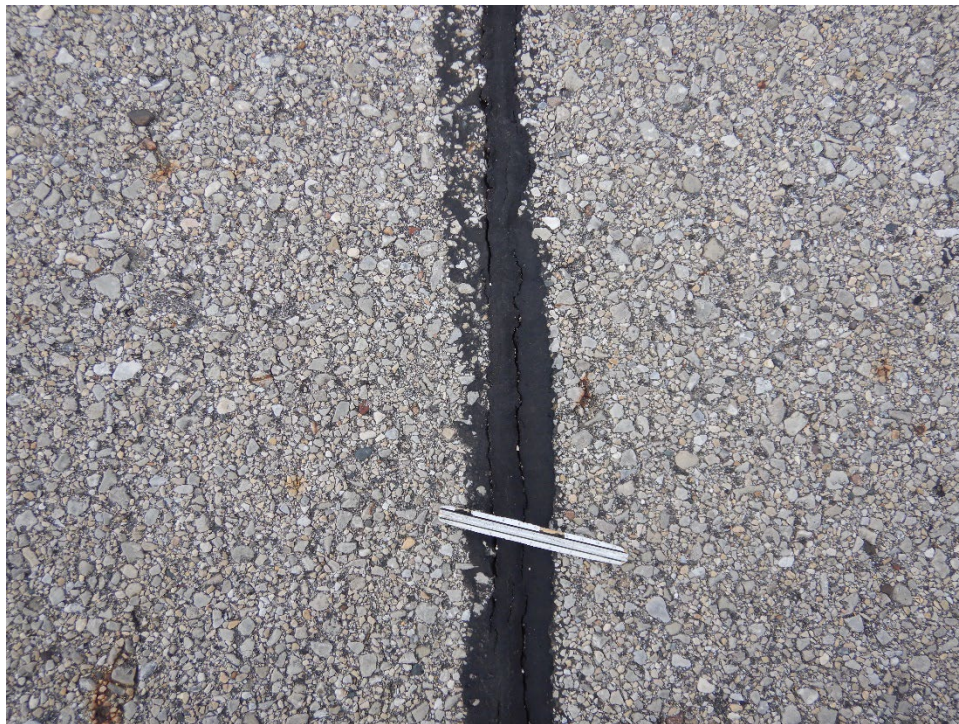
TBMC-15. L&T Cracking (Sample Unit No. 02).
