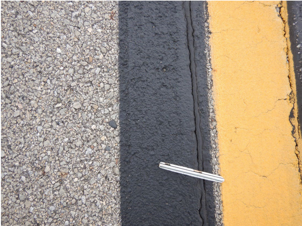
TBMC-10. L&T Cracking (Sample Unit No. 04).
