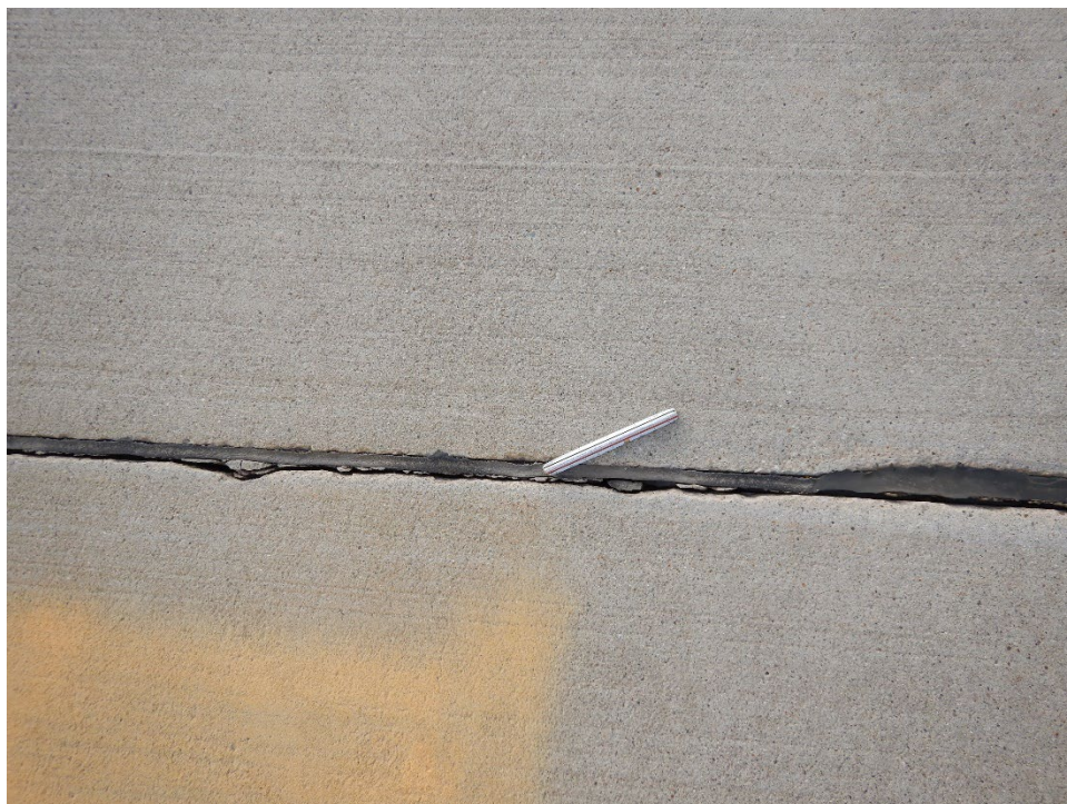
A01MC-10. Joint Seal Damage (Sample Unit No. 08).
