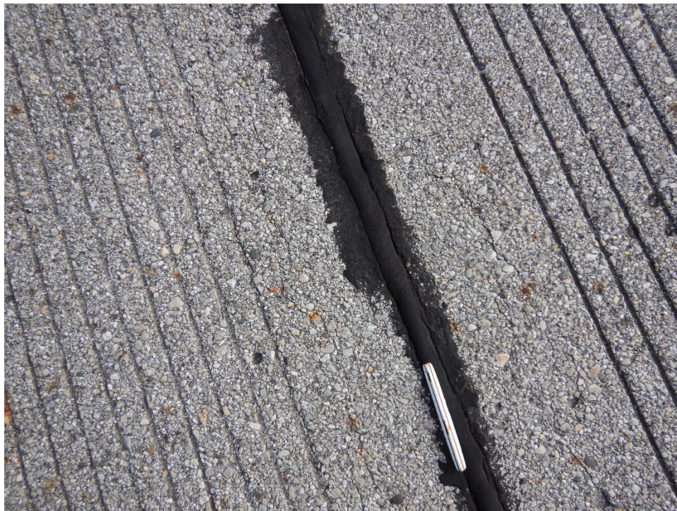
R18MC-50. L&T Cracking (Sample Unit No. 09).
