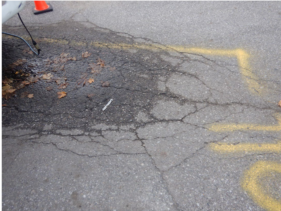
A01MC-60. Alligator Cracking (Sample Unit No. 03).
