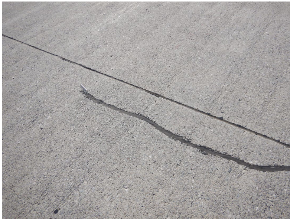
A01MC-20. Shrinkage Cracking (Sample Unit No. 05).
