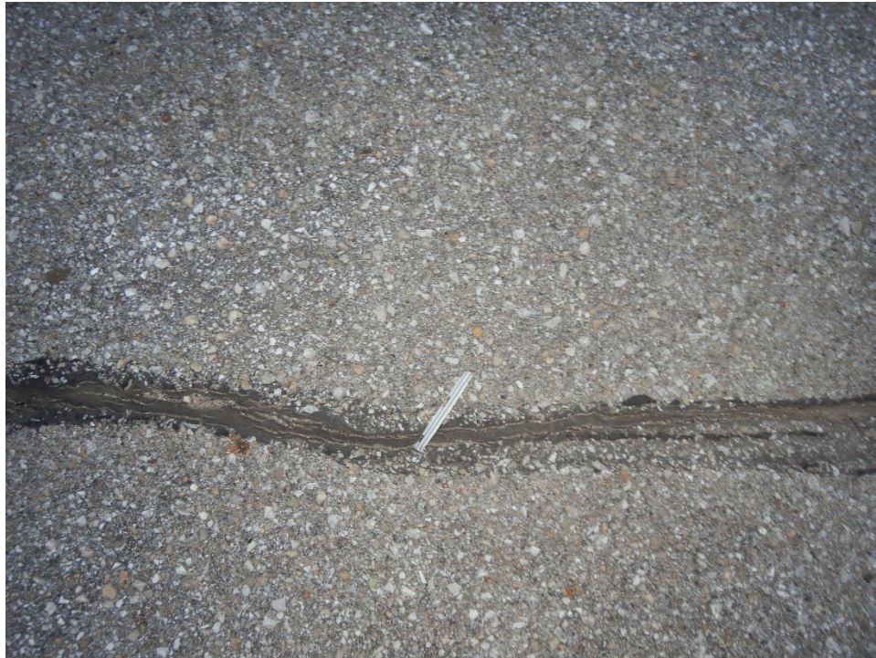
TH01MC-10. L&T Cracking (Sample Unit No. 01).
