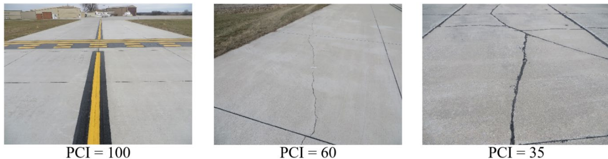
Figure 4. Visual representation of PCI scale on typical pavement surfaces 1 .
