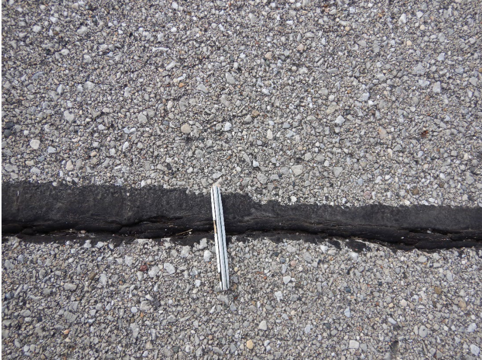
TBMC-30. L&T Cracking (Sample Unit No. 04).
