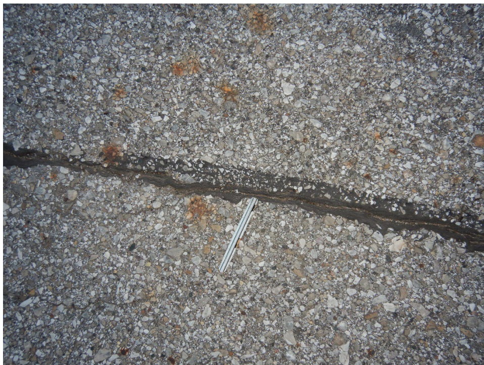
TH01MC-20. L&T Cracking (Sample Unit No. 01).
