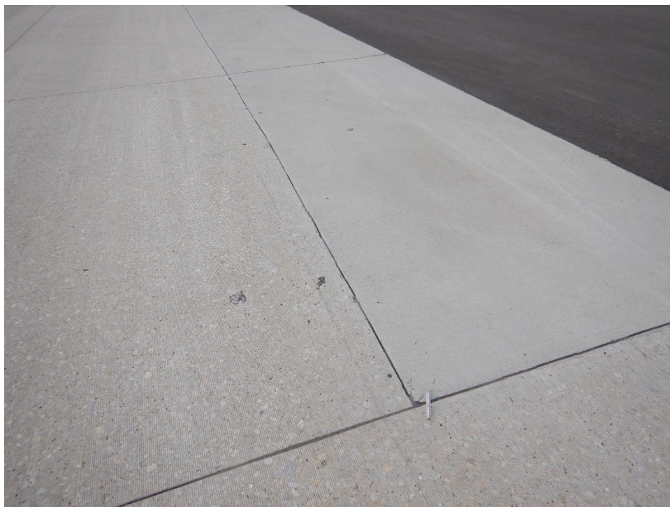
A01MC-30. Large Patching (Sample Unit No. 12).
