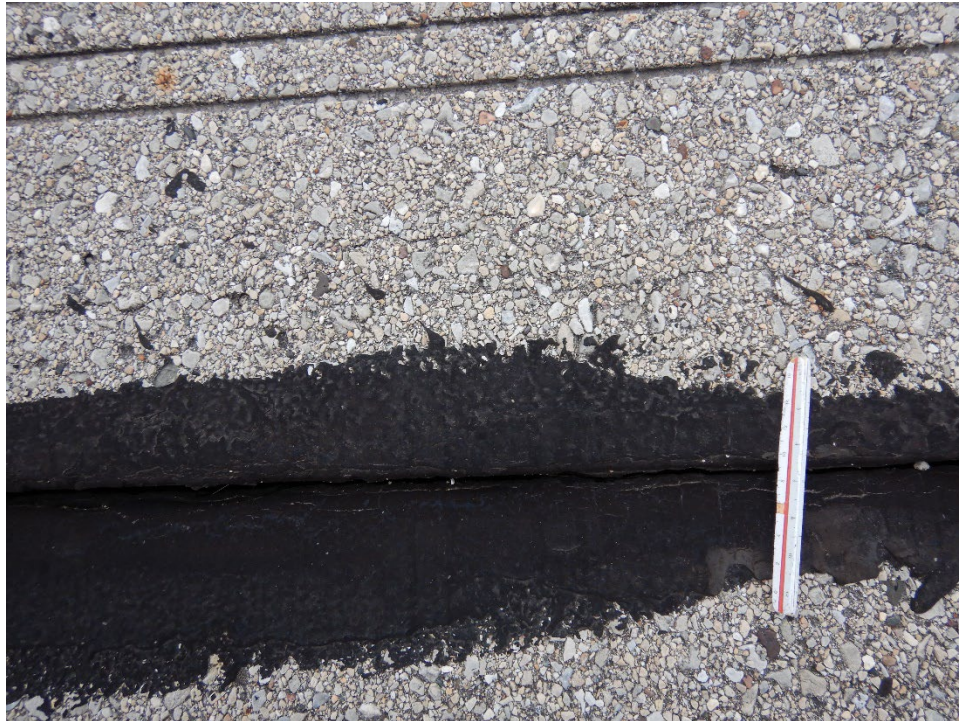
R12MC-20. L&T Cracking (Sample Unit No. 42).
