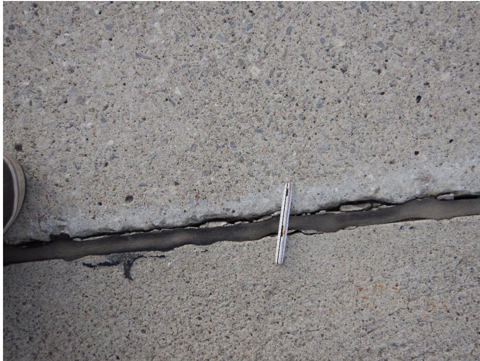
A01MC-20. Joint Seal Damage (Sample Unit No. 05).
