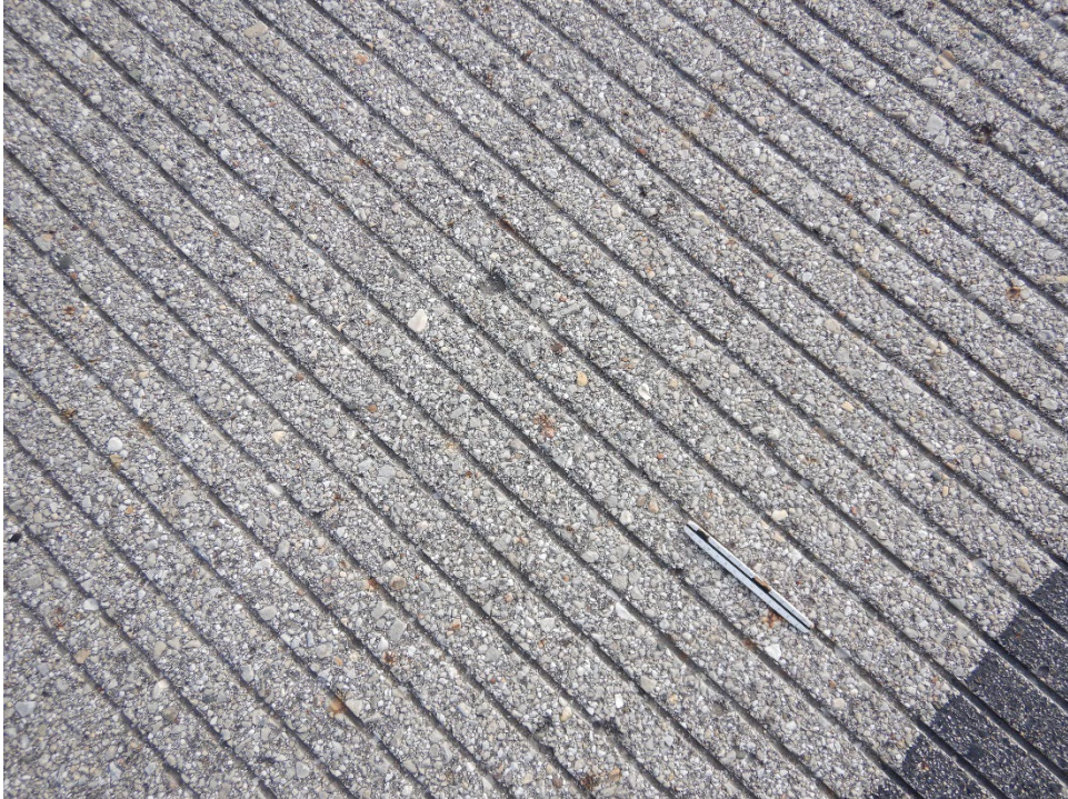
R18MC-50. Weathering (Sample Unit No. 09).
