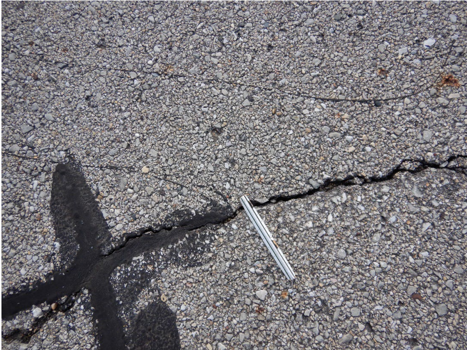
TAMC-10. L&T Cracking (Sample Unit No. 40).
