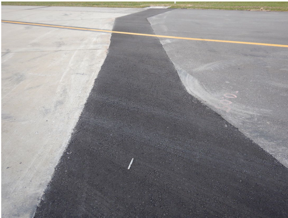
A01MC-35. Patching (Additional Sample Unit No. 13).
