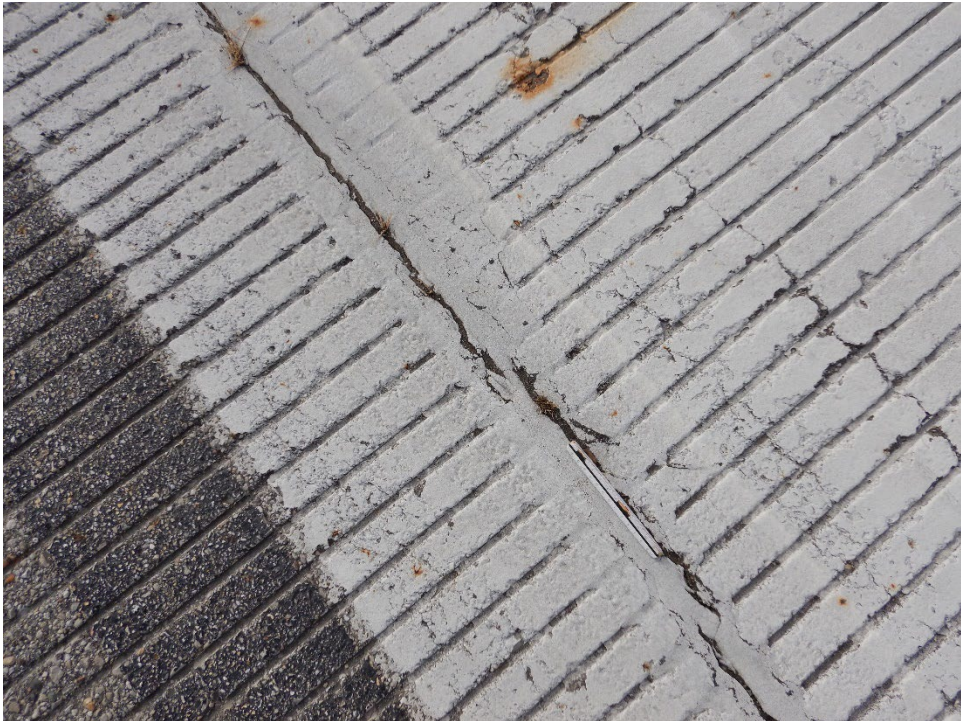
R18MC-60. L&T Cracking (Sample Unit No. 09).
