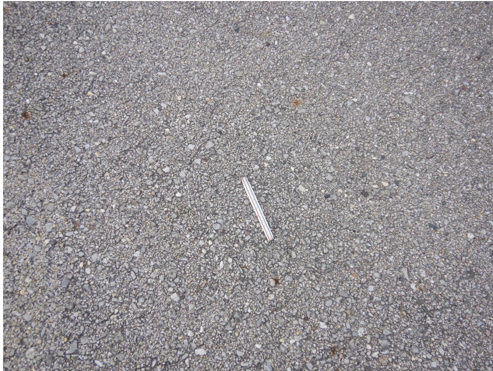
TBMC-35. Weathering (Sample Unit No. 02).
