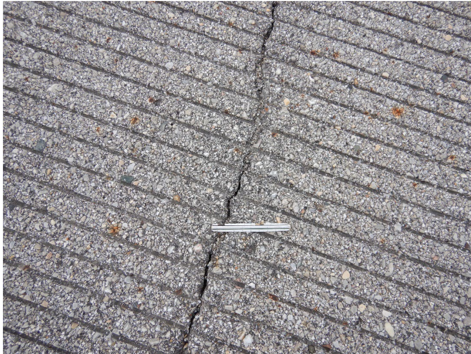
R12MC-40. L&T Cracking (Sample Unit No. 01).
