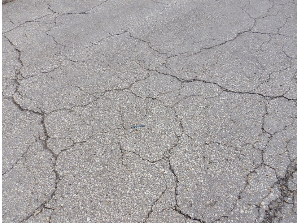
TH02MT-01. Block Cracking (Sample Unit No. 01).
