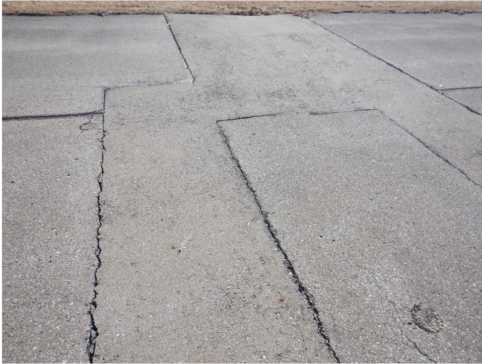
R18MT-02. Patching (Sample Unit No. 03).
