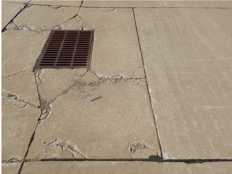
TH01MT-01. Large Patching (Additional Sample Unit No. 07).
