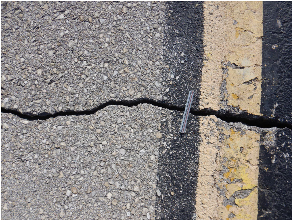
T03MT-01. L&T Cracking (Sample Unit No. 03).
