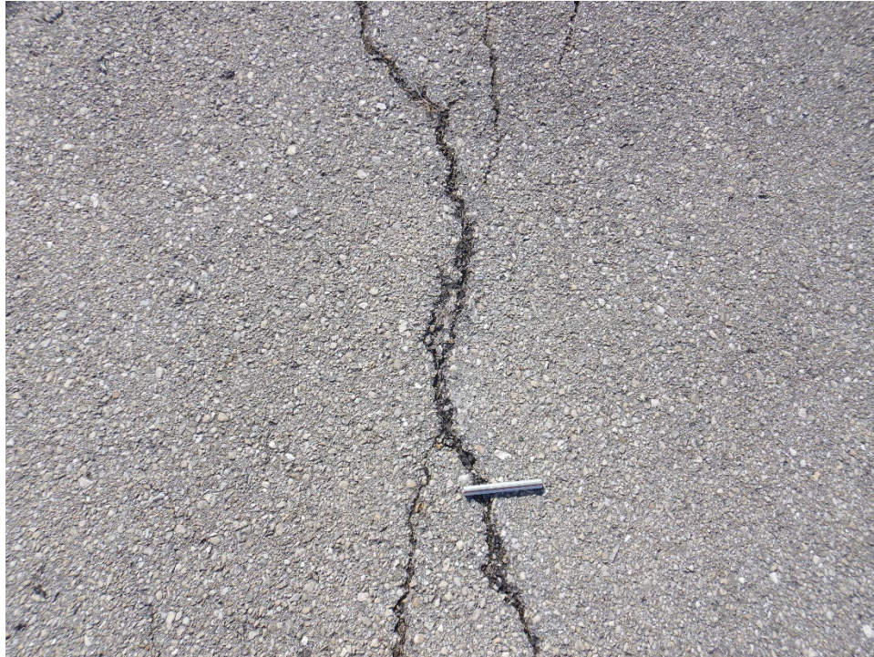
T03MT-02. L&T Cracking (Sample Unit No. 01).
