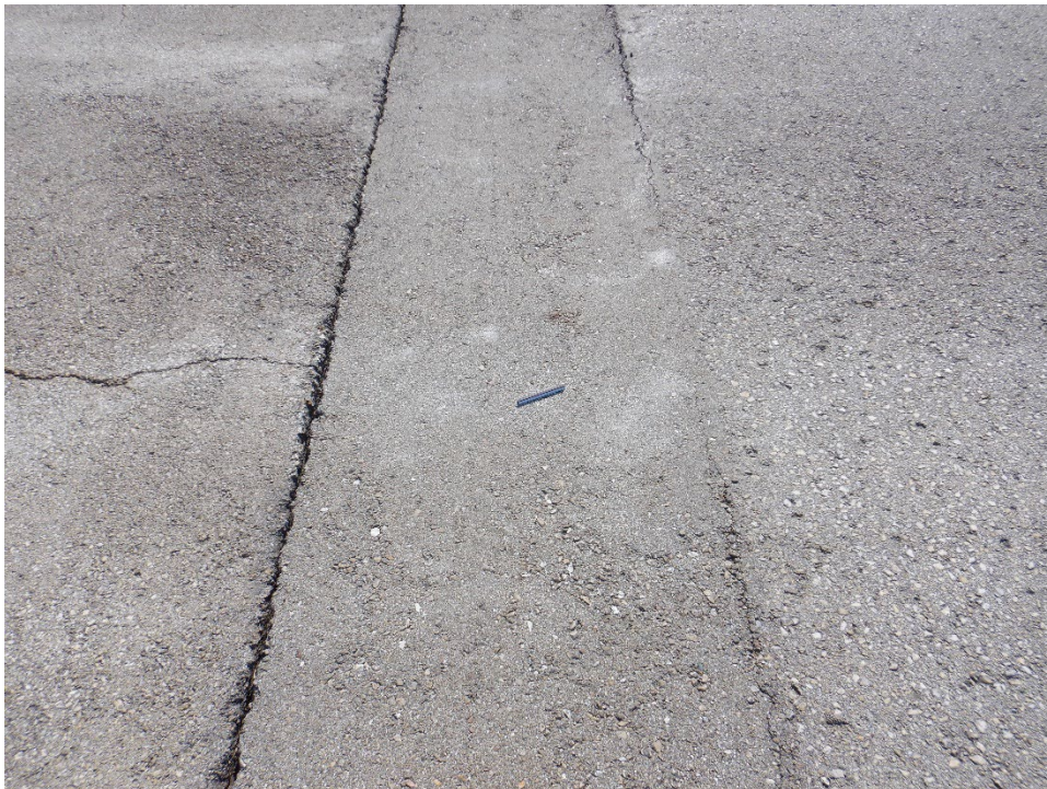
R13MT-03. Patching (Sample Unit No. 01).
