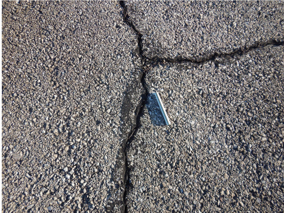
R18MT-04. L&T Cracking (Sample Unit No. 02).
