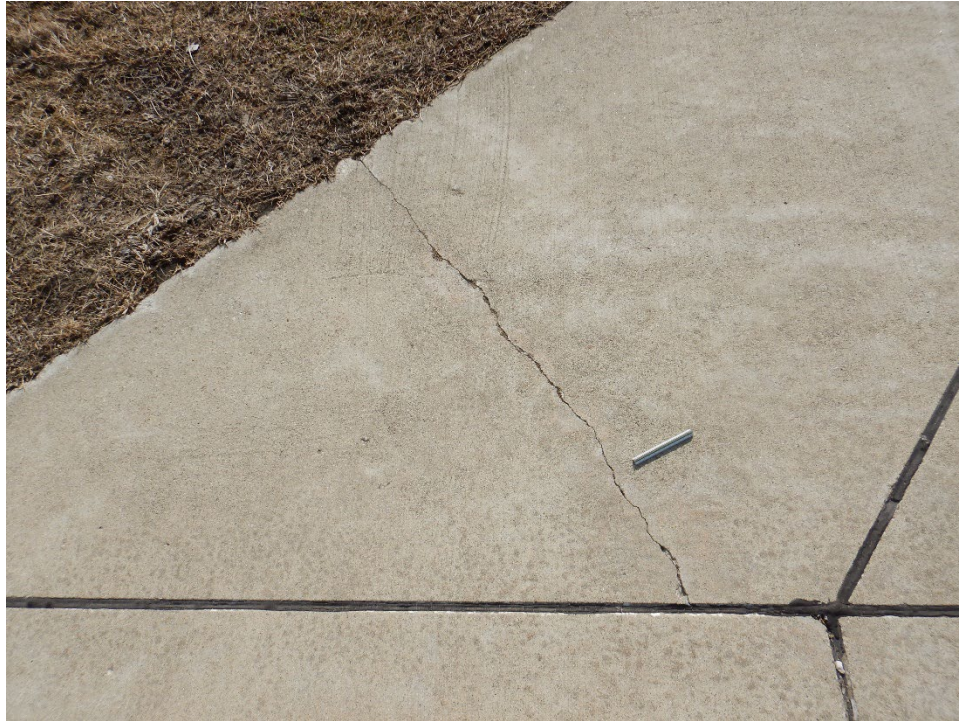
TH01MT-01. LTD Cracking (Additional Sample Unit No. 04).
