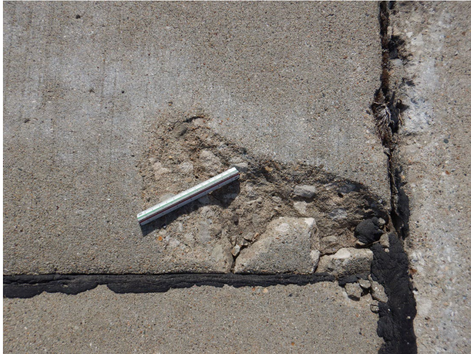
A02MT-01. Corner Spalling (Sample Unit No. 18).
