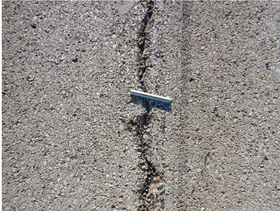
R13MT-01. L&T Cracking (Sample Unit No. 19) (2).
