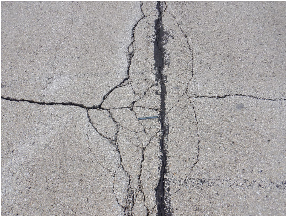
T02MT-01. Alligator Cracking (Sample Unit No. 05).
