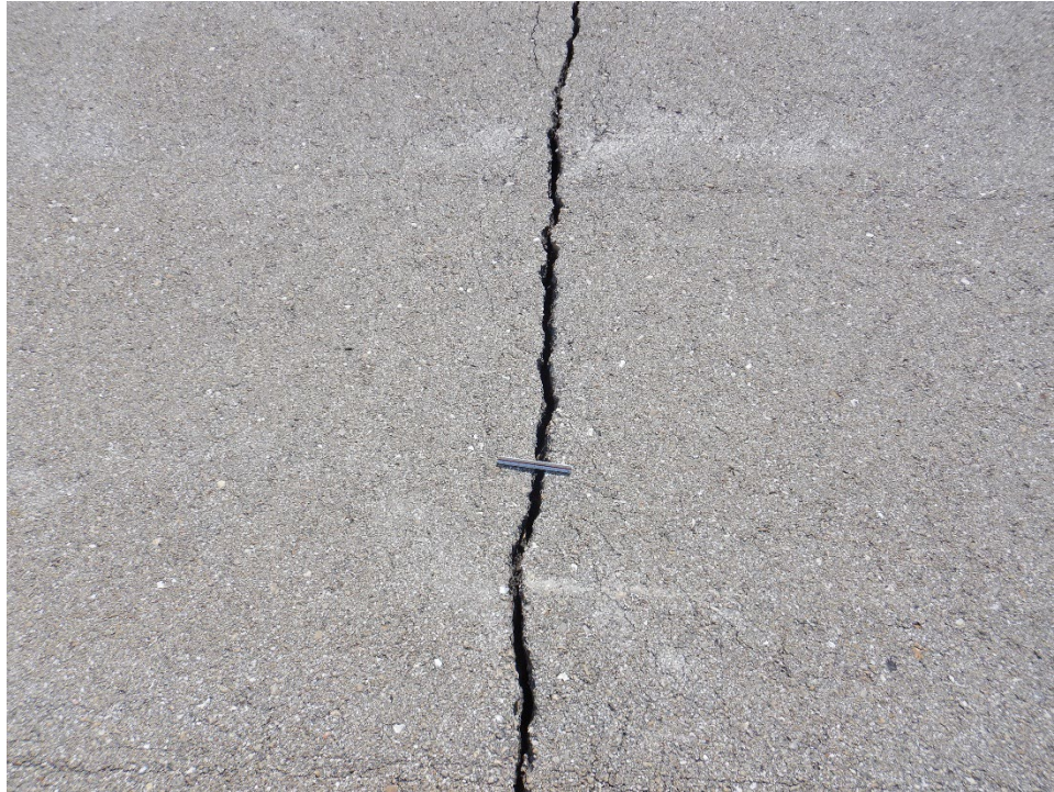
T01MT-01. L&T Cracking (Sample Unit No. 02).
