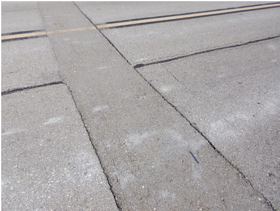
T04MT-01. Patching (Sample Unit No. 05).
