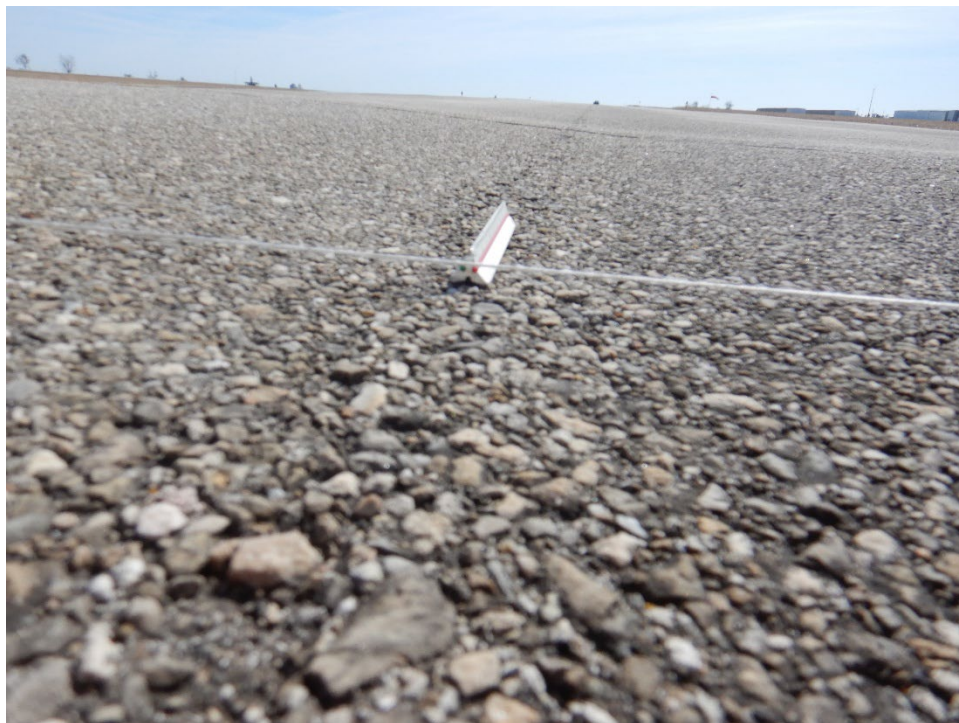
T03MT-03. Rutting (Additional Sample Unit No. 05).
