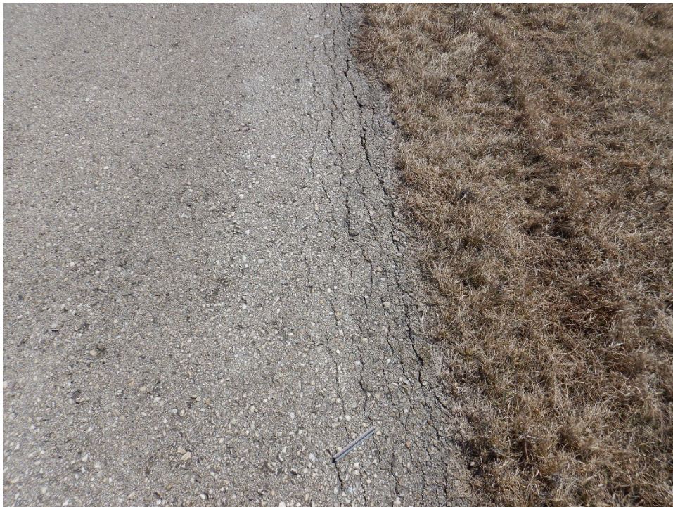
T04MT-01. Alligator Cracking (Sample Unit No. 05) (1).
