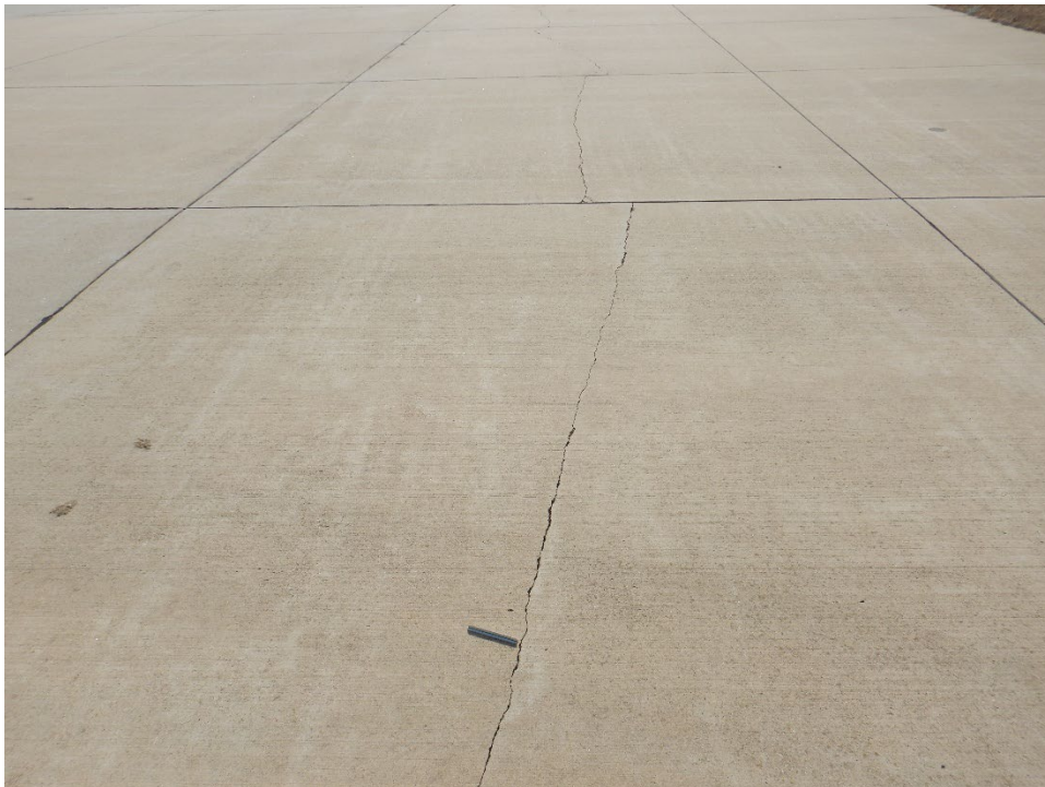
TH01MT-02. LTD Cracking (Sample Unit No. 05).
