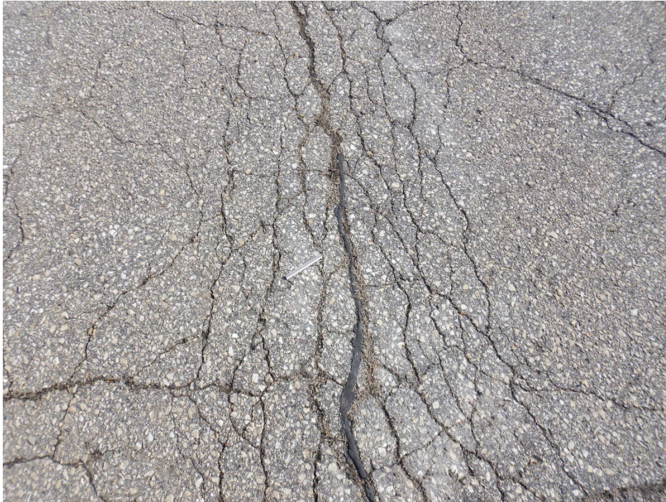
A02MT-02. Alligator Cracking (Sample Unit No. 02).
