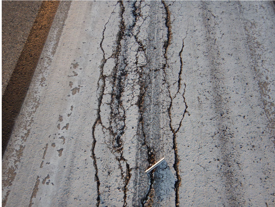
R13MT-02. Alligator Cracking (Sample Unit No. 75).
