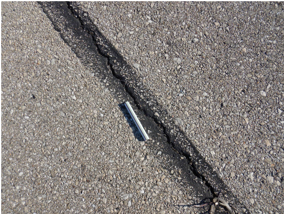
R18MT-02. L&T Cracking (Sample Unit No. 03).
