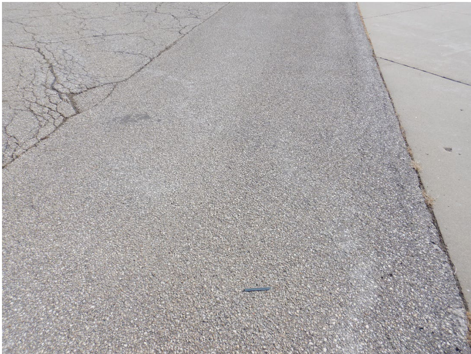
A02MT-02. Patching (Sample Unit No. 02).
