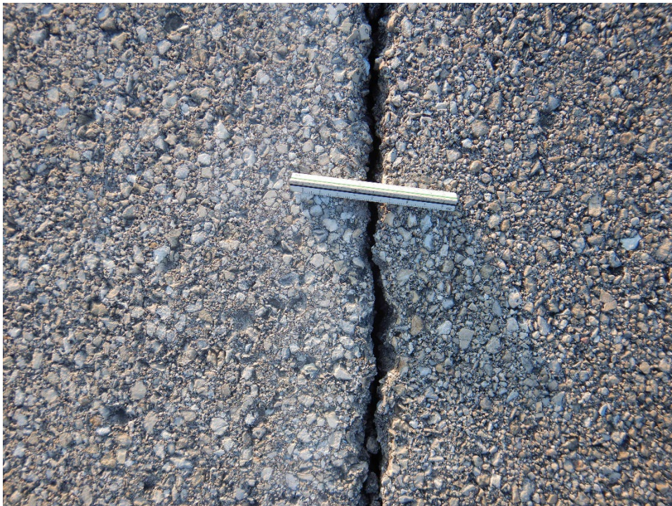
R13MT-02. L&T Cracking (Sample Unit No. 75).
