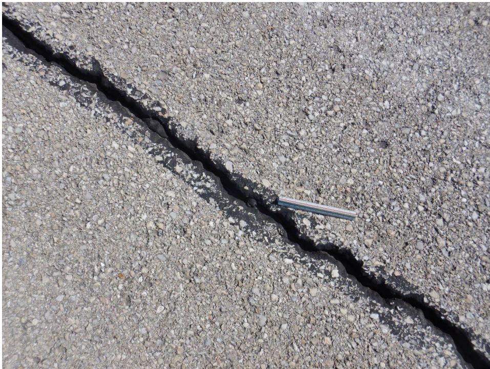
T02MT-02. L&T Cracking (Sample Unit No. 01).
