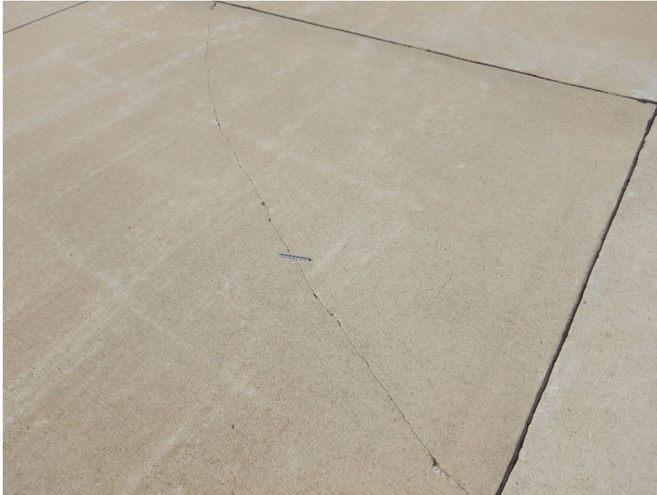
TH01MT-02. LTD Cracking (Sample Unit No. 02).
