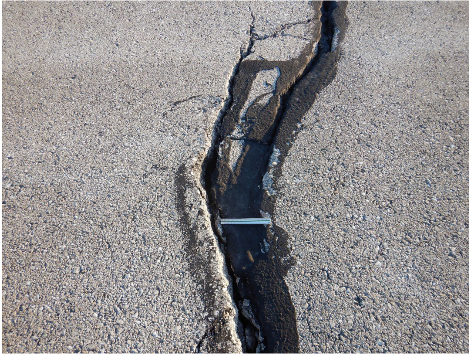
R13MT-02. L&T Cracking (Sample Unit No. 65).
