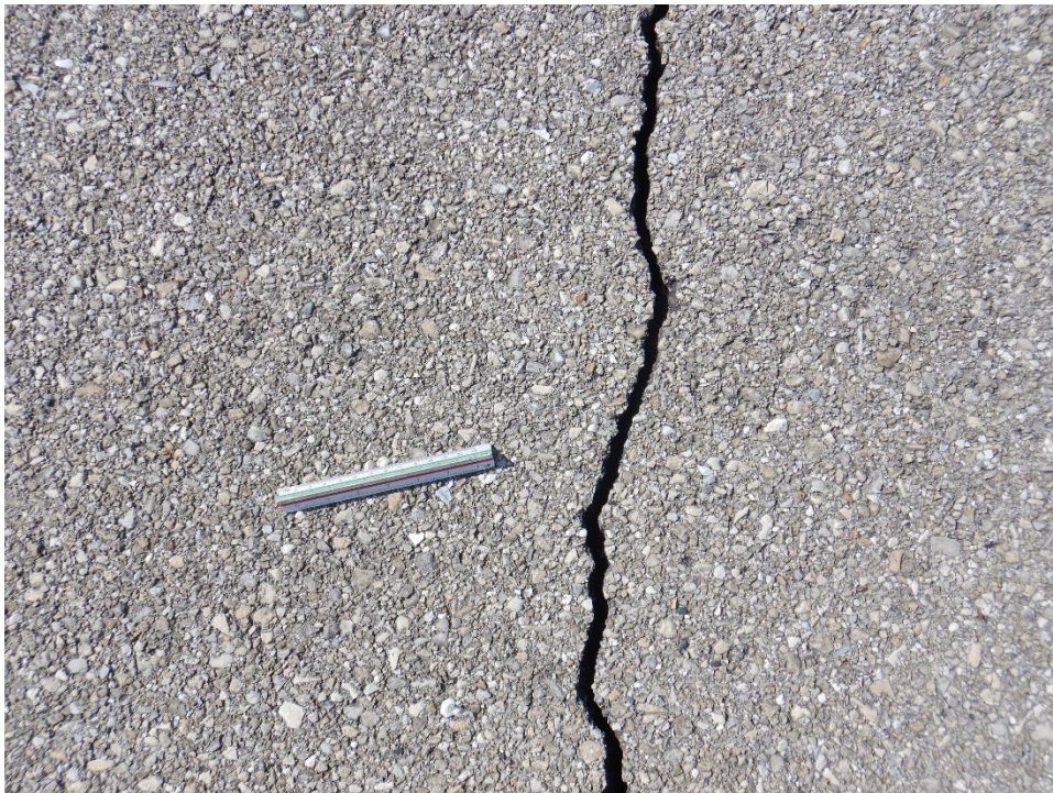
T03MT-03. L&T Cracking (Sample Unit No. 04).
