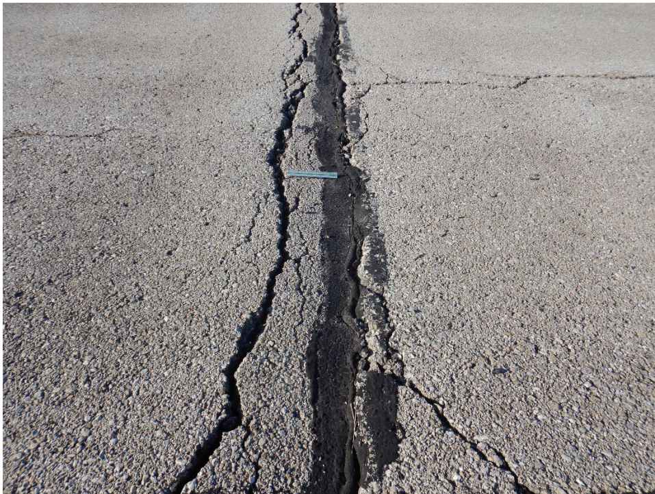
R13MT-01. L&T Cracking (Sample Unit No. 19) (1).
