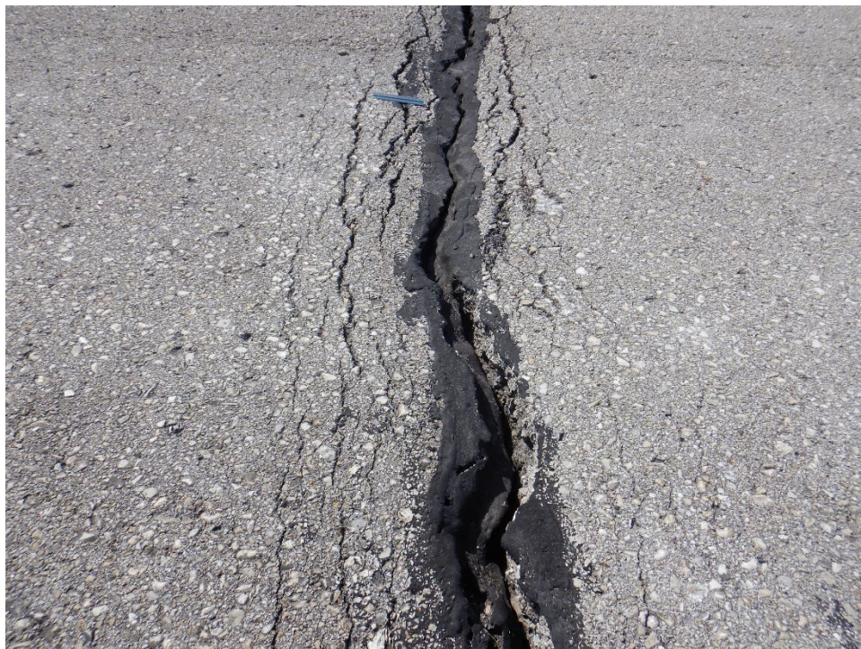
T04MT-01. L&T Cracking (Sample Unit No. 03).
