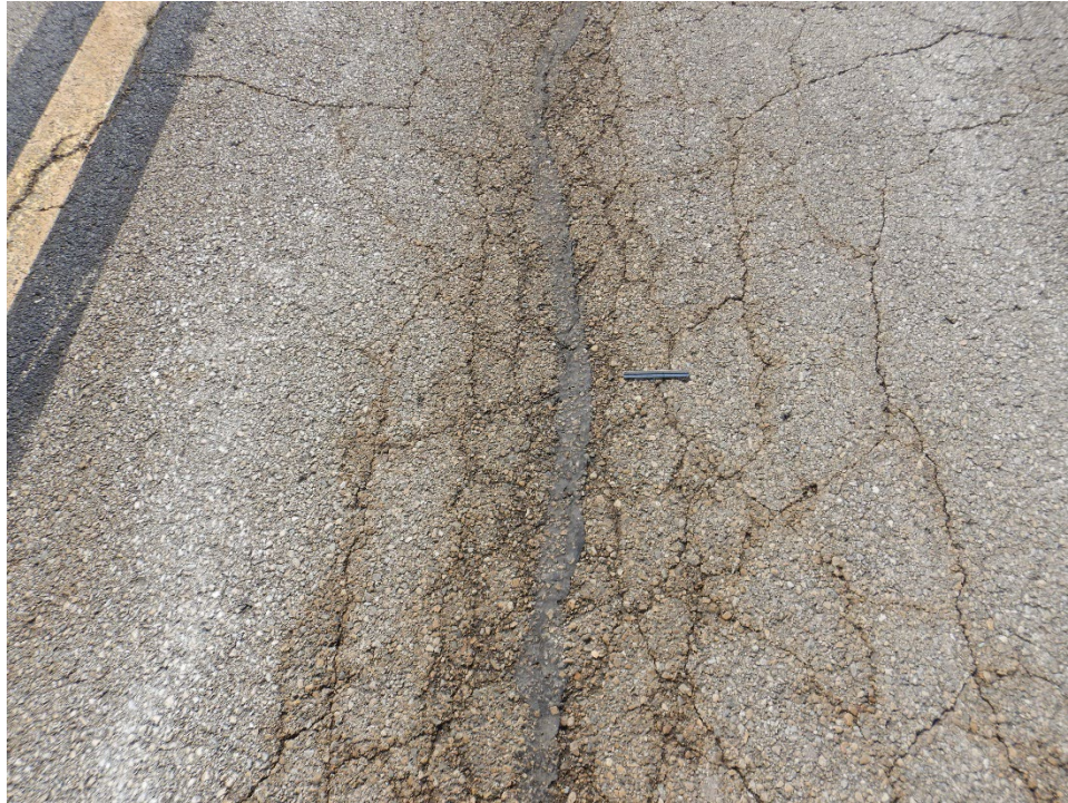
R13MT-04. Alligator Cracking (Sample Unit No. 02).
