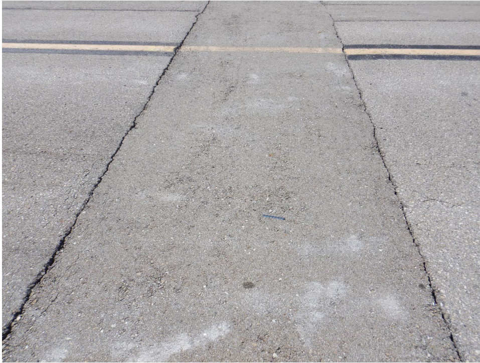
T04MT-01. Patching (Sample Unit No. 03).
