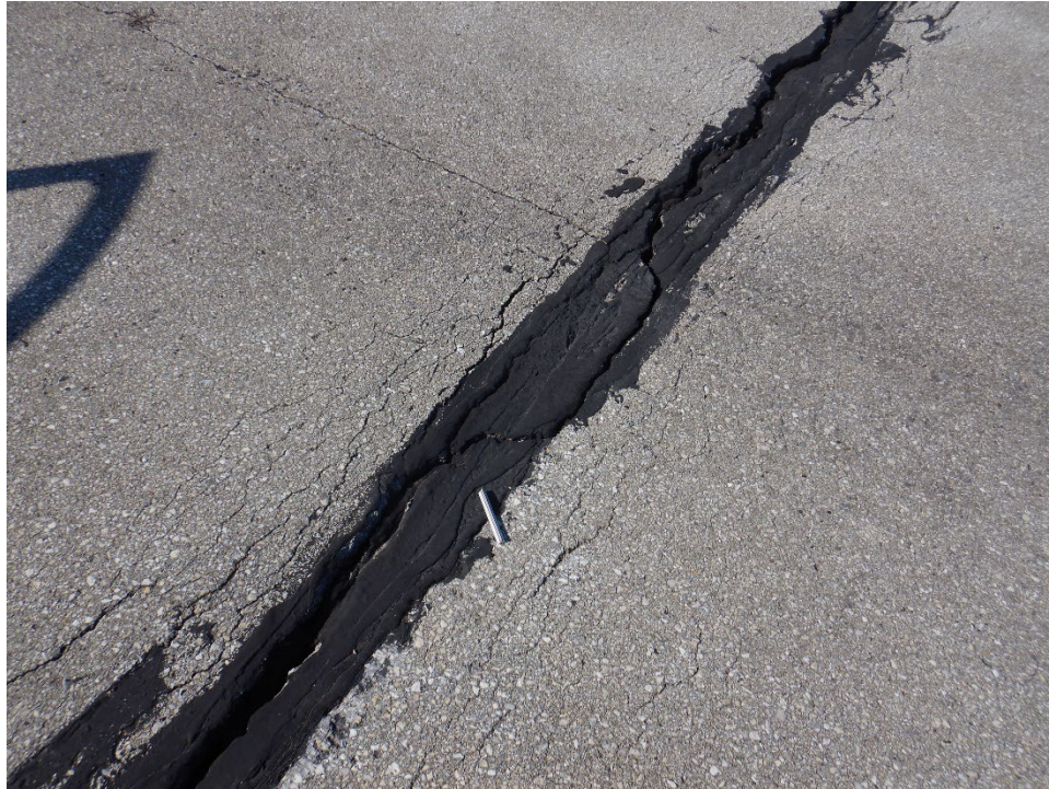
R18MT-01. L&T Cracking (Sample Unit No. 10).
