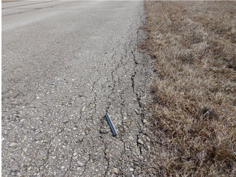
T04MT-01. Alligator Cracking (Sample Unit No. 05) (2).
