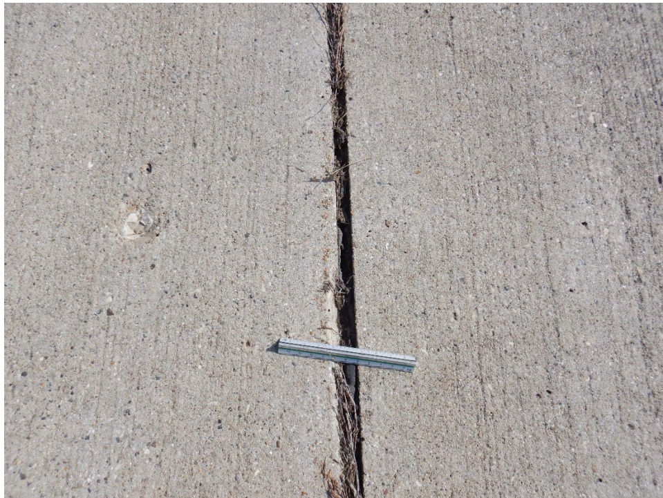
A01MT-01. Joint Seal Damage (Sample Unit No. 04).
