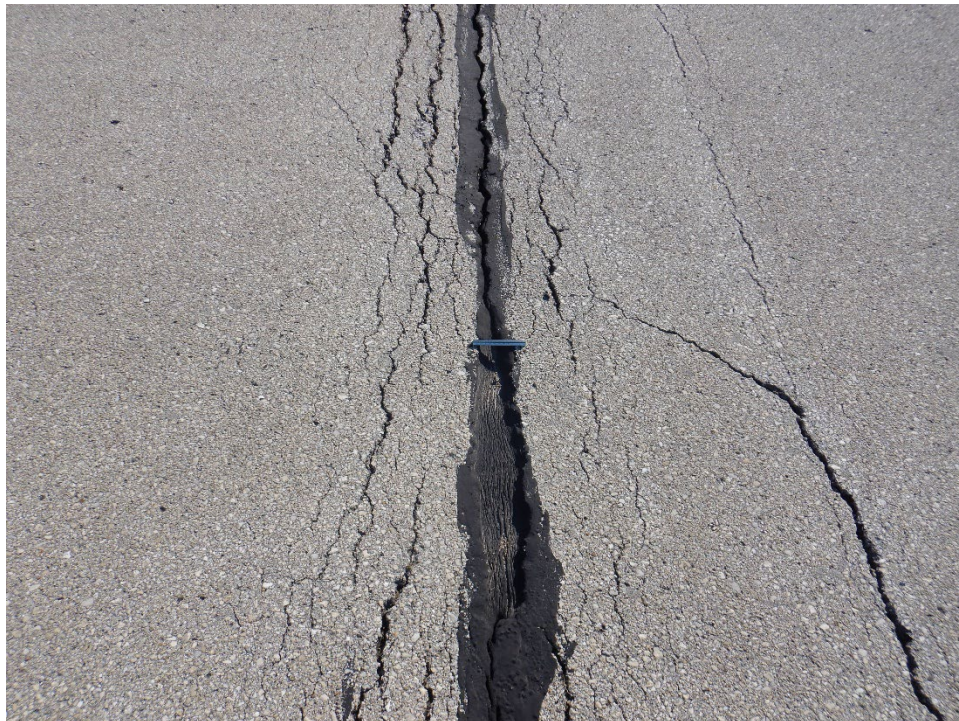
R18MT-01. L&T Cracking (Sample Unit No. 18).
