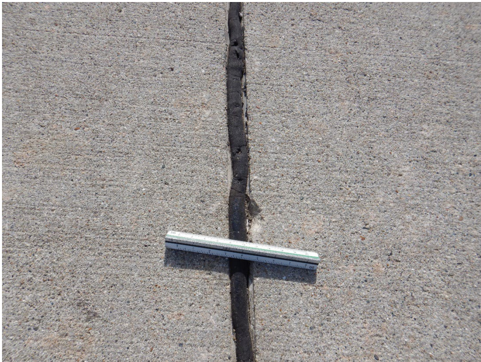
A03MT-01. Joint Seal Damage (Sample Unit No. 04).
