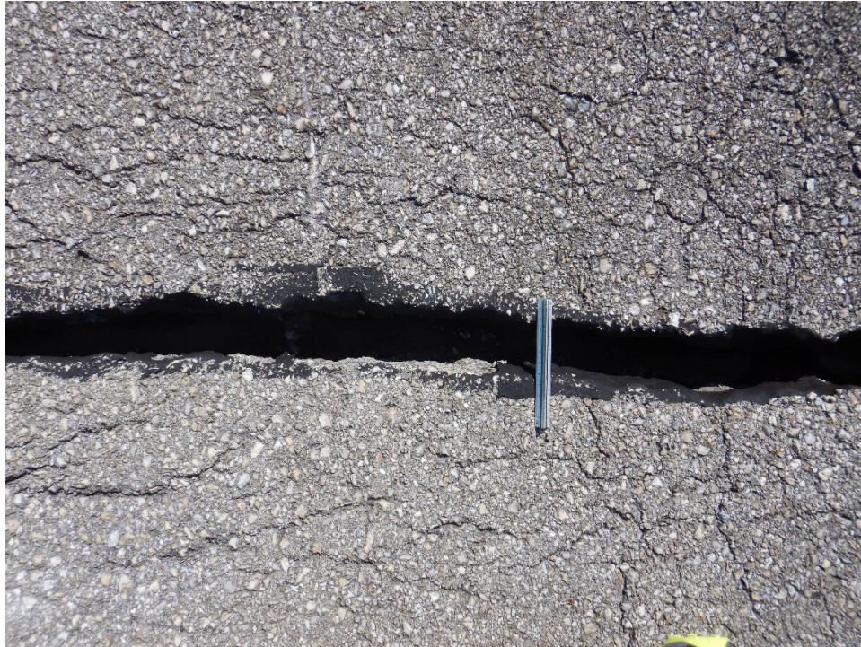
T03MT-03. L&T Cracking (Sample Unit No. 08).
