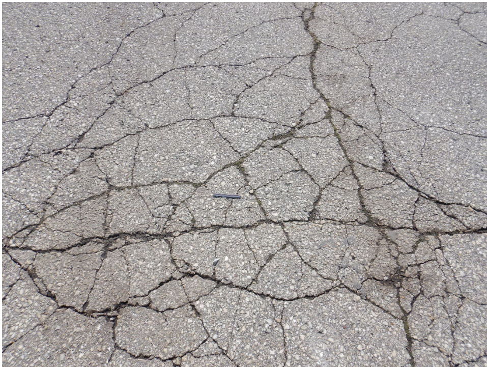
TH02MT-01. Alligator Cracking (Sample Unit No. 01).
