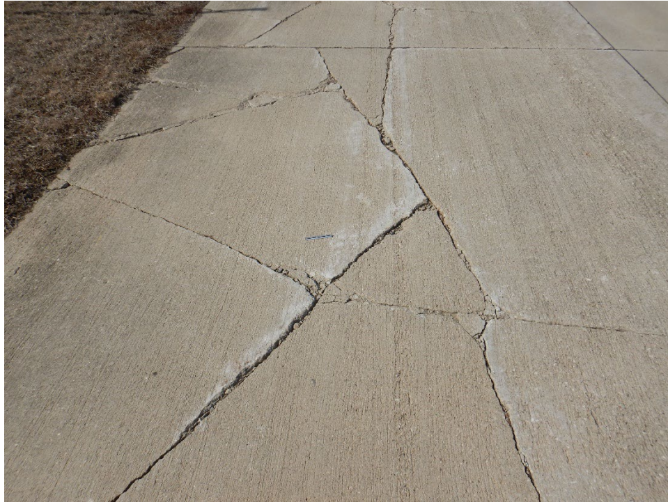
A01MT-01. Shattered Slab (Additional Sample Unit No. 23).
