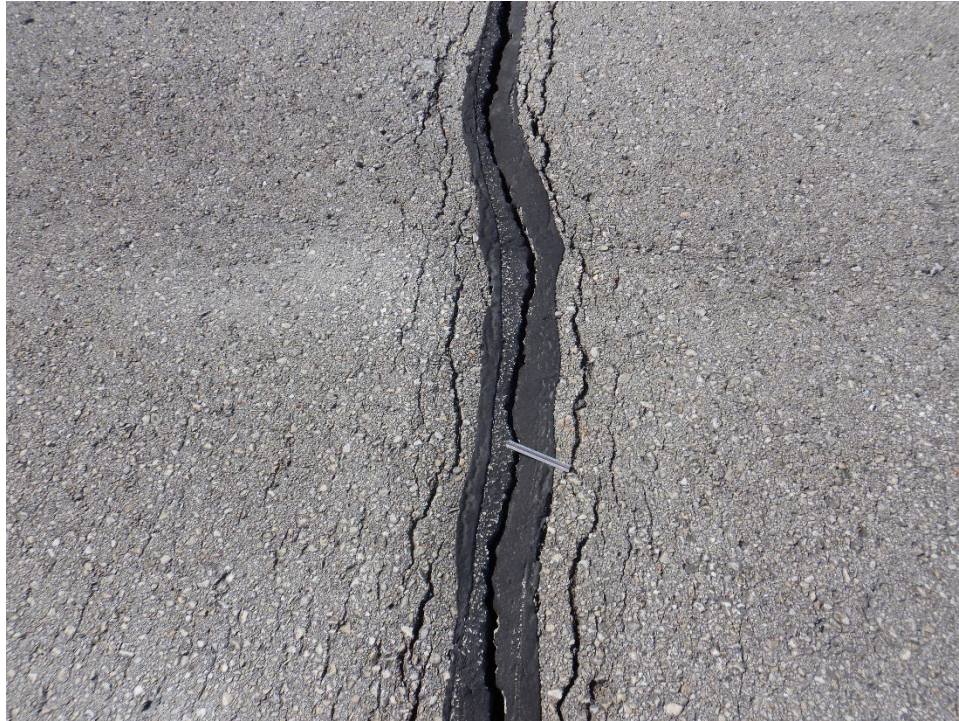
T03MT-01. L&T Cracking (Sample Unit No. 10).
