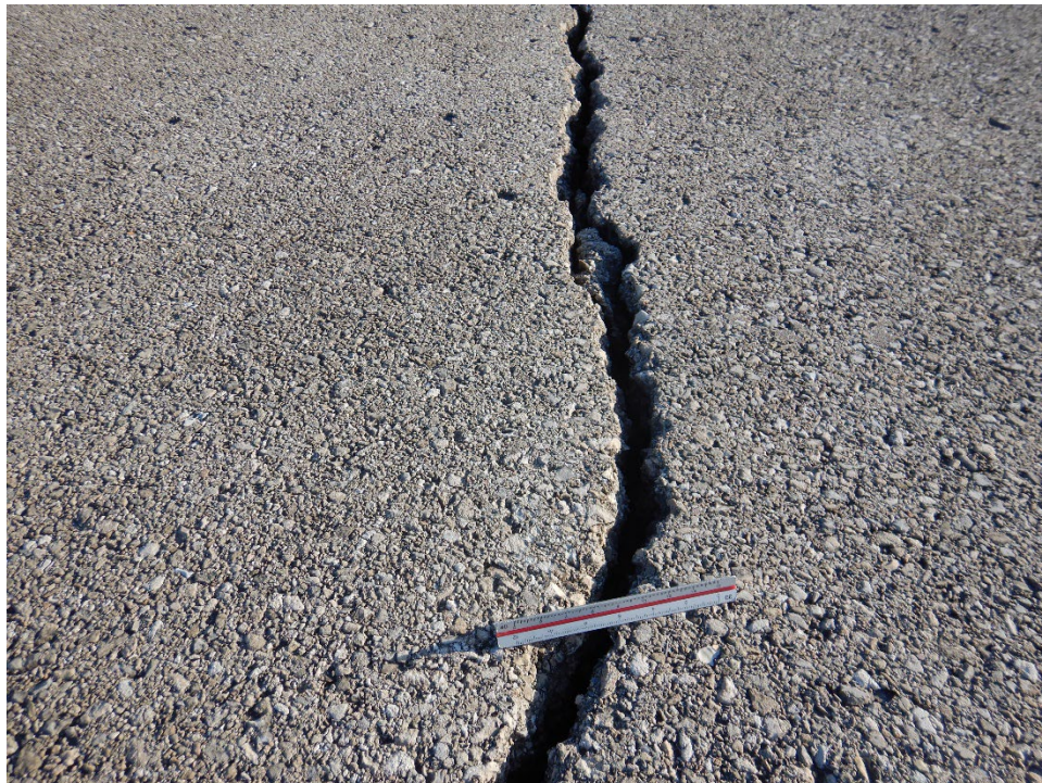
R13MT-02. L&T Cracking (Sample Unit No. 15).
