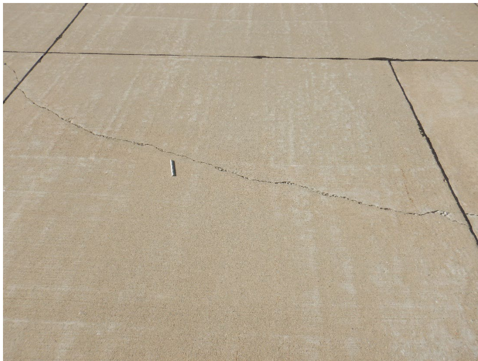
TH01MT-01. LTD Cracking (Additional Sample Unit No. 07).
