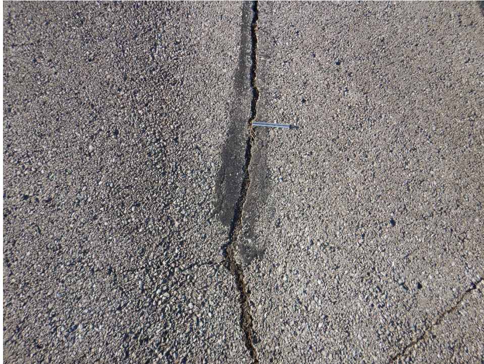
R18MT-03. L&T Cracking (Sample Unit No. 02).
