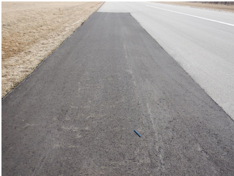
R17MR-02. Patching (Additional Sample Unit No. 08).
