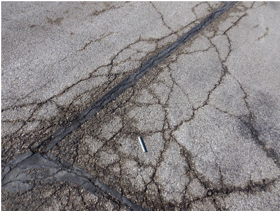
A01MR-01. Alligator Cracking (Sample Unit No. 05).
