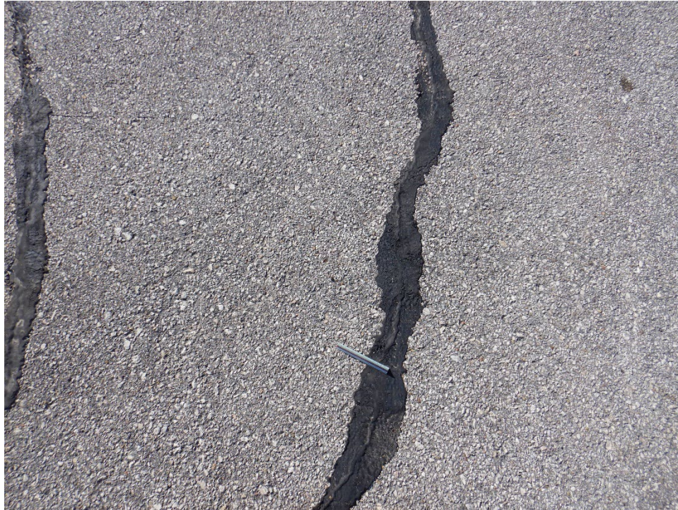
A01MR-02. L&T Cracking (Sample Unit No. 02).
