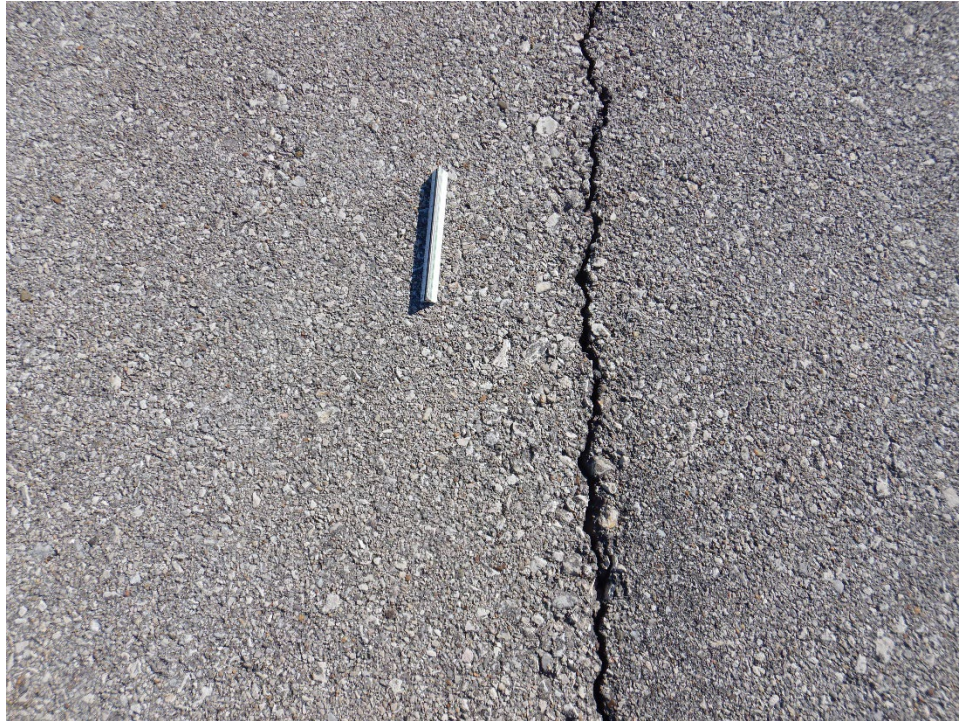
T01MR-01. L&T Cracking (Sample Unit No. 01).
