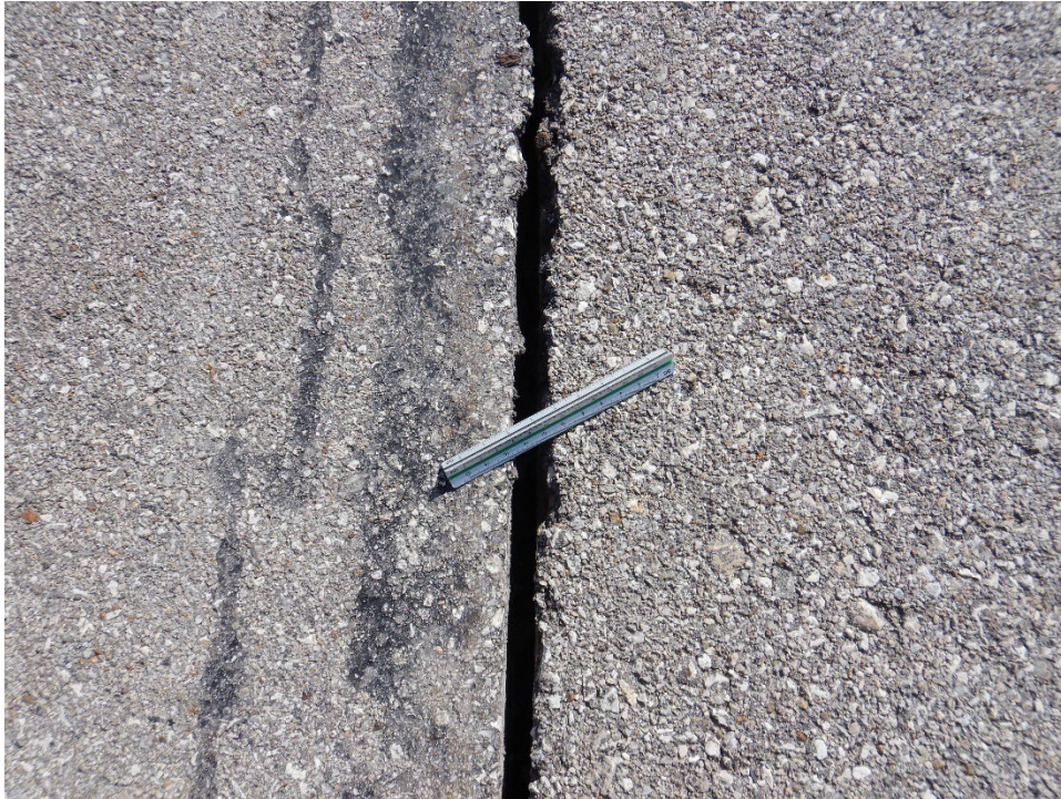
R17MR-04. L&T Cracking (Sample Unit No. 04).
