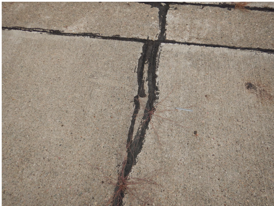
R02MA-01. Joint Spalling (Sample Unit No. 17).
