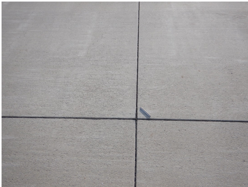
TH01MA-01. Joint Seal Damage (Sample Unit No. 04).
