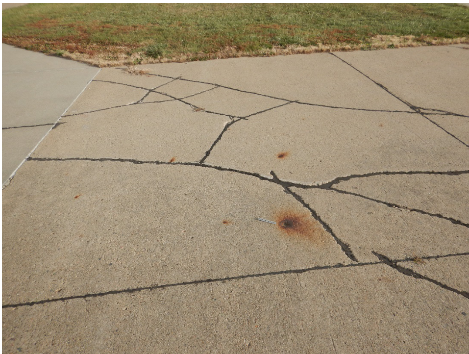
A01MA-01. Shattered Slab (Sample Unit No. 01).
