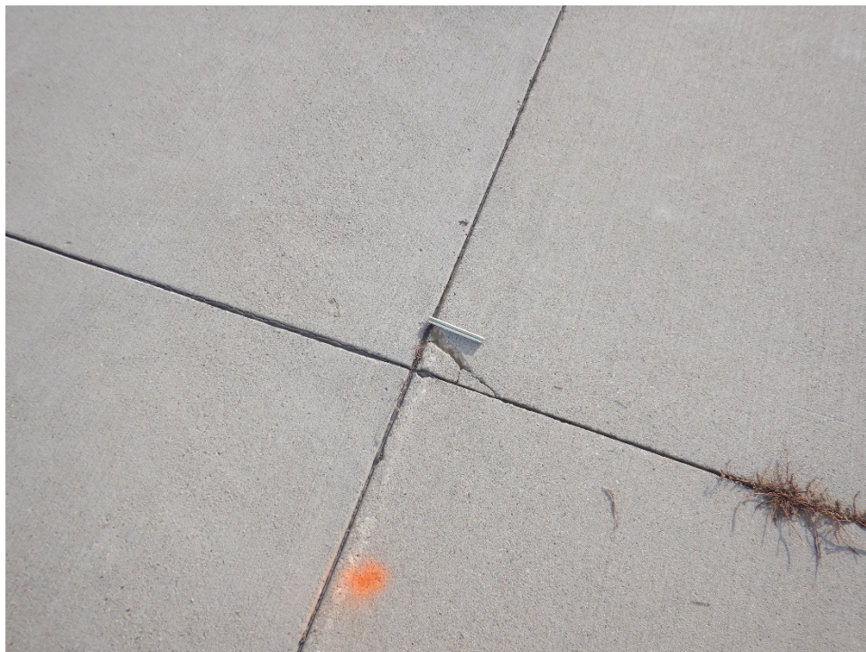
TH01MA-02. Corner Spalling (Sample Unit No. 10).
