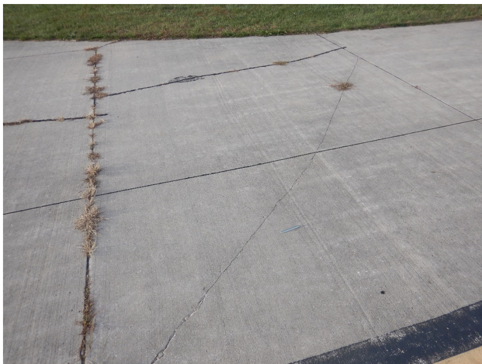
T03MA-01. LTD Cracking (Sample Unit No. 02).
