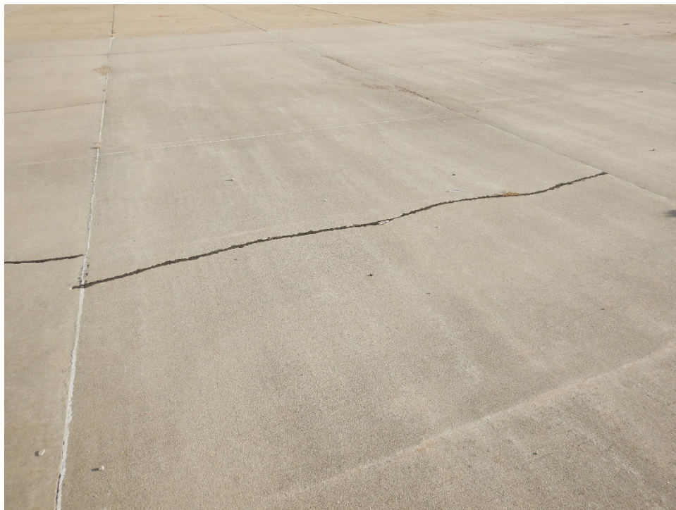
A01MA-03. LTD Cracking (Sample Unit No. 02).
