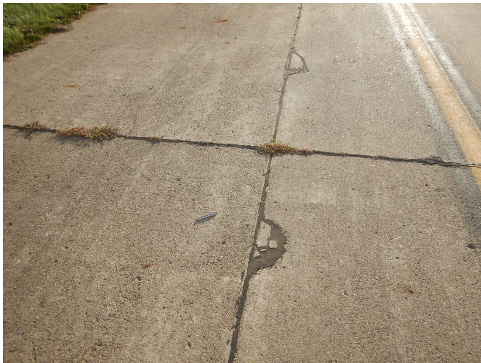
T01MA-01. Joint Spalling (Sample Unit No. 02).
