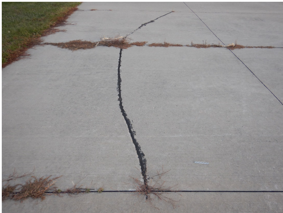
T02MA-01. LTD Cracking (Sample Unit No. 02).
