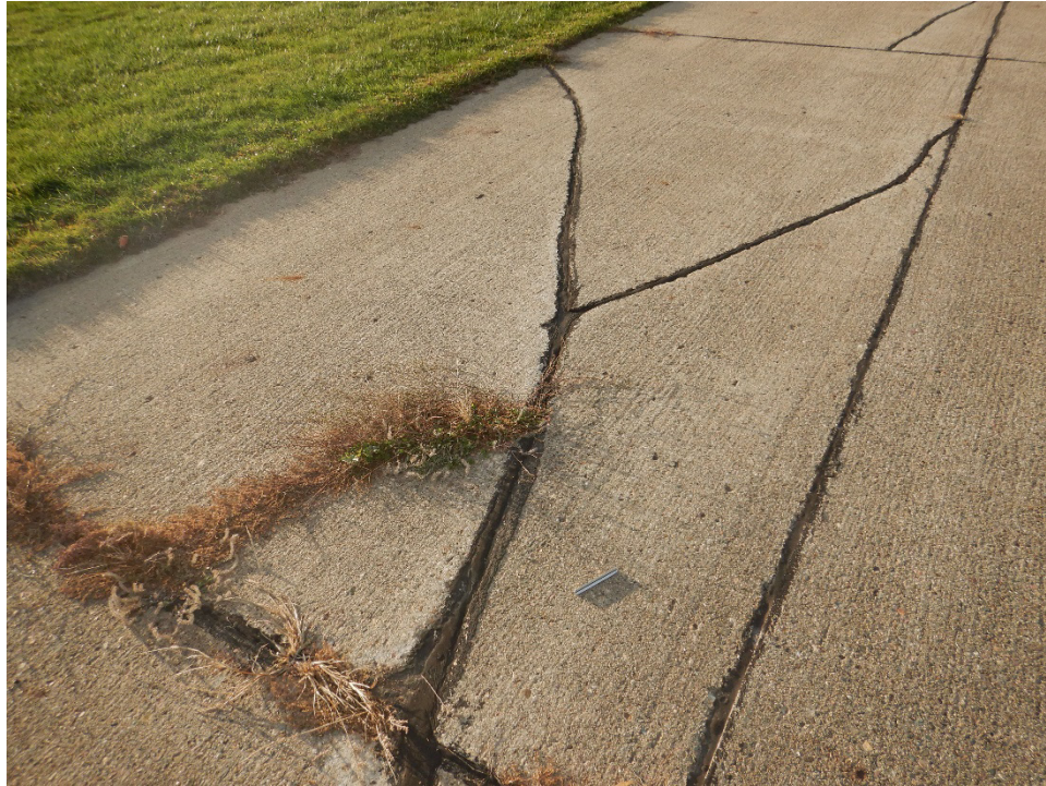
R02MA-01. Shattered Slab (Sample Unit No. 22).
