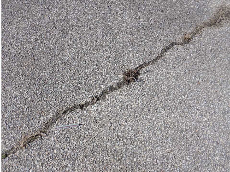
TH01C2-01. L&T Cracking (Sample Unit No. 01).
