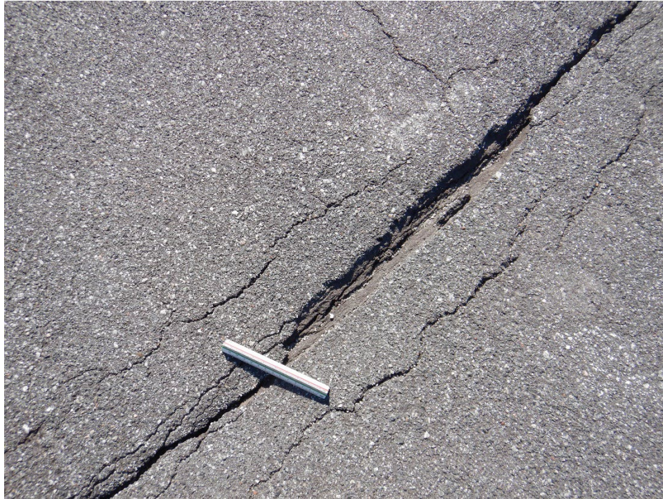
T01C2-02. L&T Cracking (Sample Unit No. 01).
