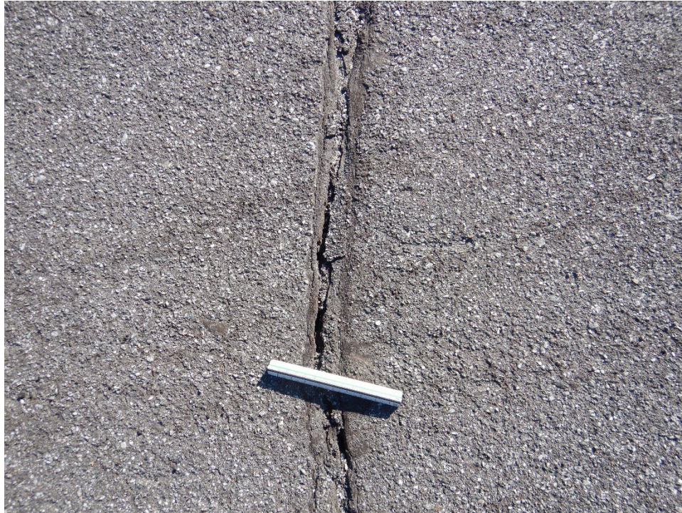
R18C2-02. L&T Cracking (Sample Unit No. 01).
