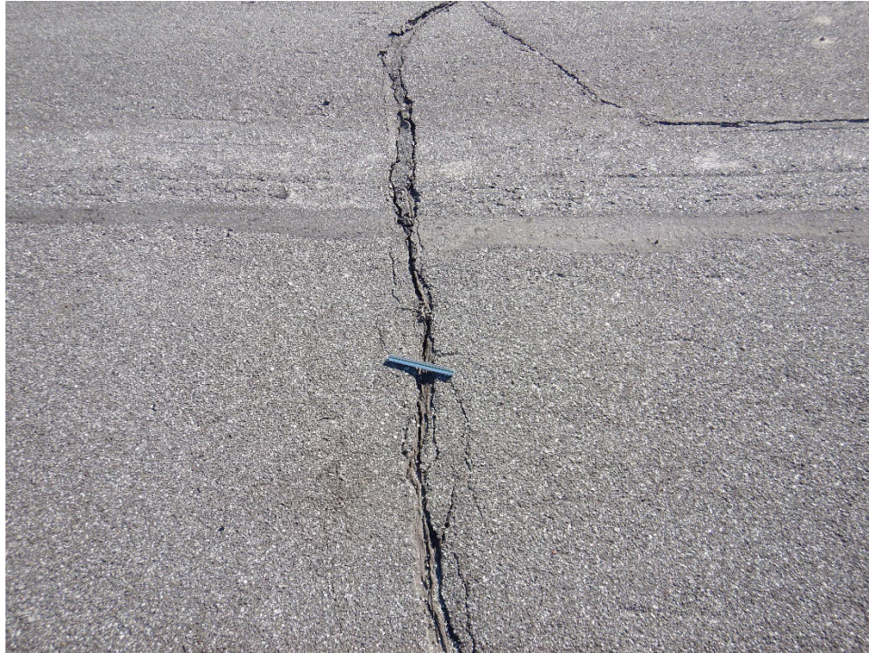
R18C2-01. L&T Cracking (Sample Unit No. 03).
