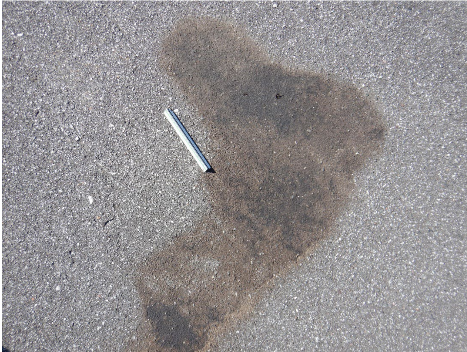
A02C2-03. Oil-Fuel Damage (Sample Unit No. 05).
