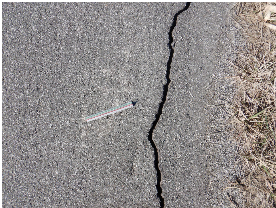
A02C2-03. L&T Cracking (Sample Unit No. 06) (2).
