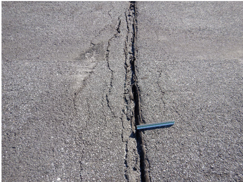
R18C2-01. L&T Cracking (Sample Unit No. 11).
