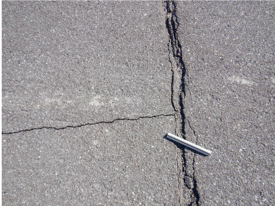
A02C2-02. L&T Cracking (Sample Unit No. 01).
