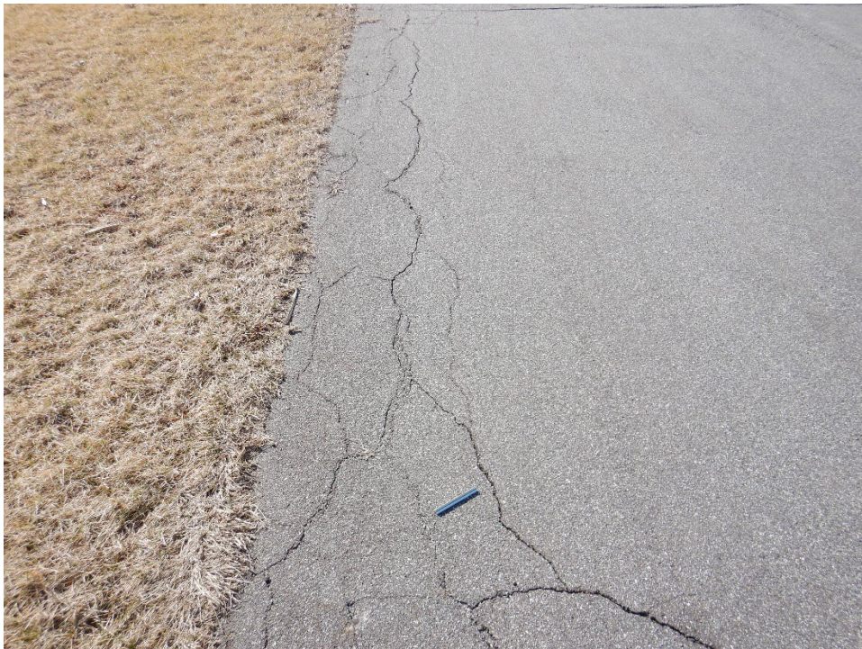
R18C2-01. Alligator Cracking (Sample Unit No. 27).
