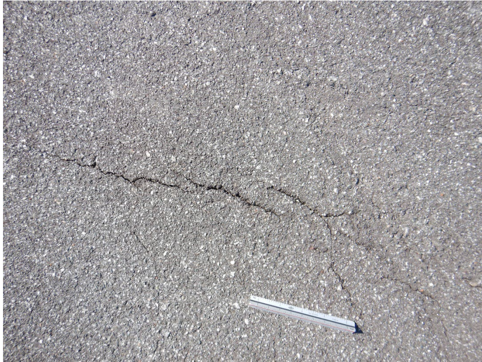
A02C2-03. L&T Cracking (Sample Unit No. 06) (1).
