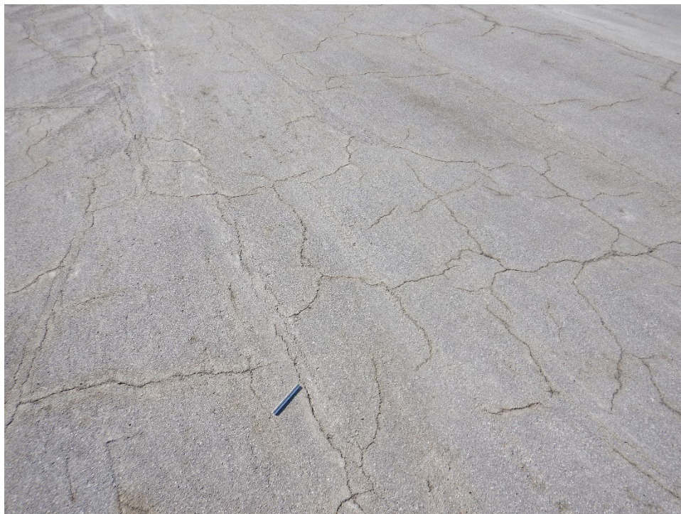
A01C2-01. Block Cracking (Sample Unit No. 01).
