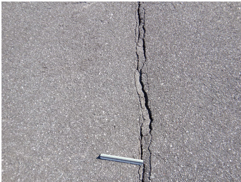
A02C2-01. L&T Cracking (Sample Unit No. 01).
