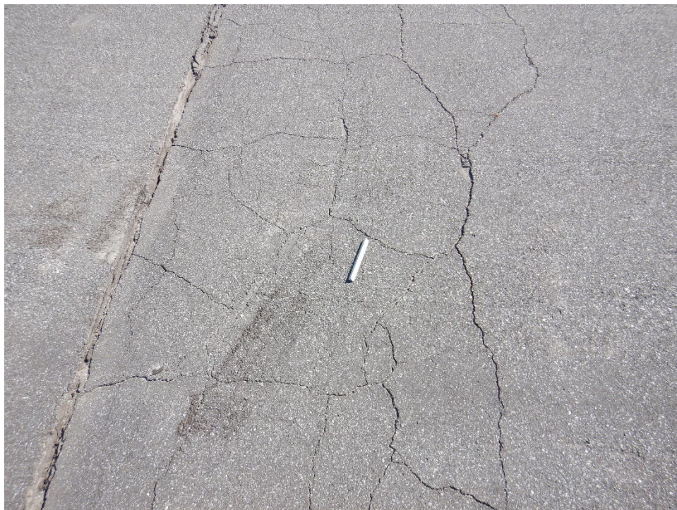
A02C2-02. Alligator Cracking (Sample Unit No. 02).
