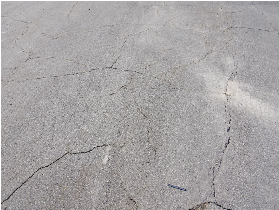
T01C2-01. Block Cracking (Sample Unit No. 02).
