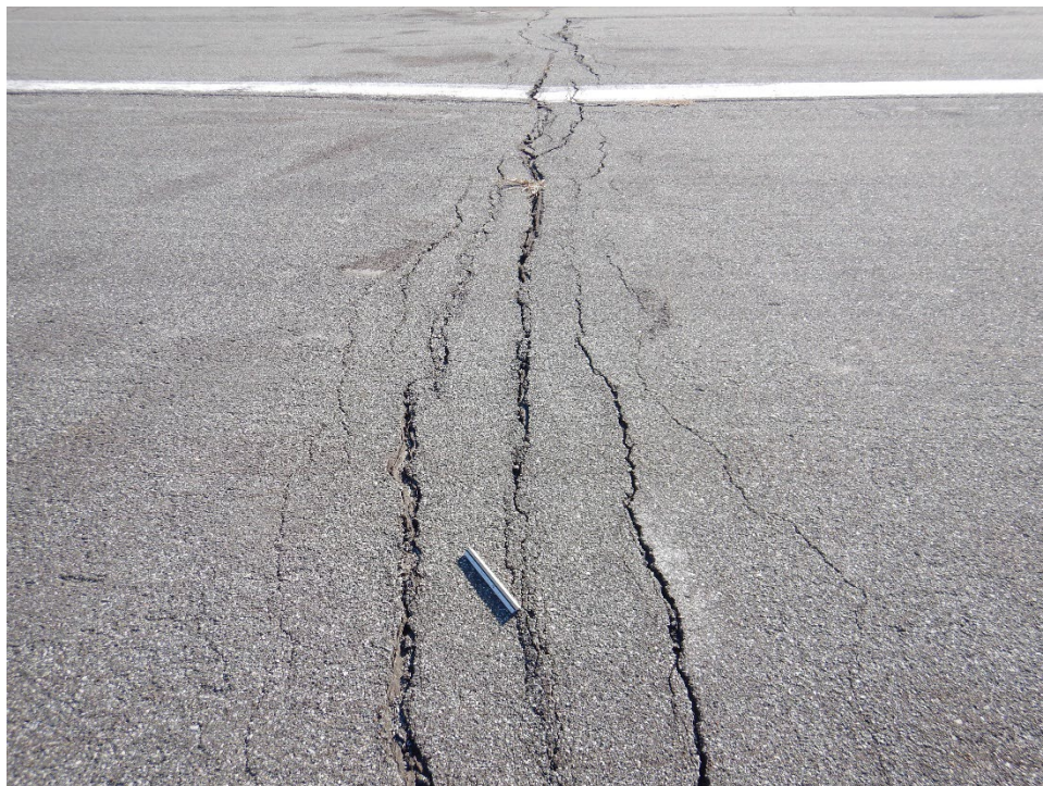
R18C2-02. L&T Cracking (Sample Unit No. 05).
