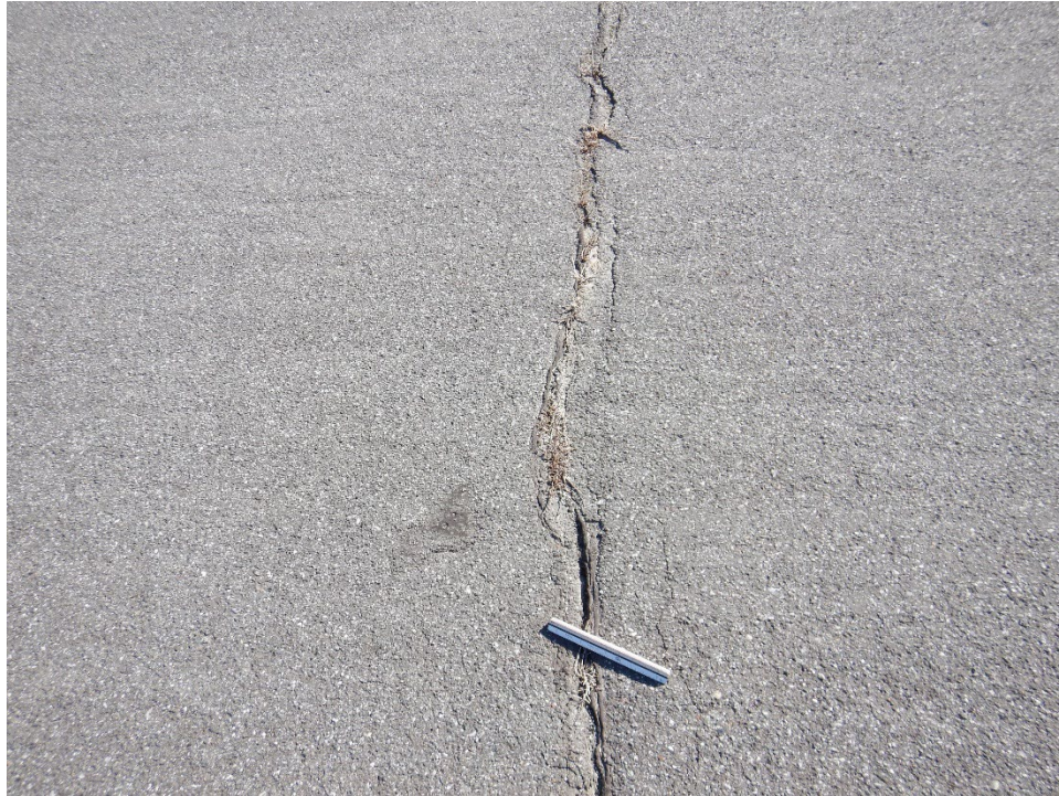
T01C2-01. L&T Cracking (Sample Unit No. 02).
