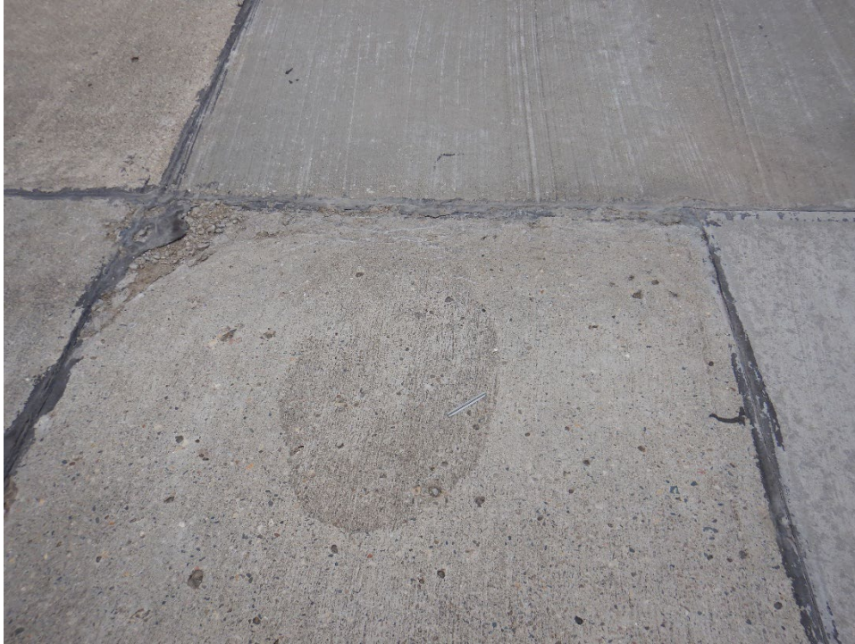
A01LE-02. Durability Cracking (Sample Unit No. 05).
