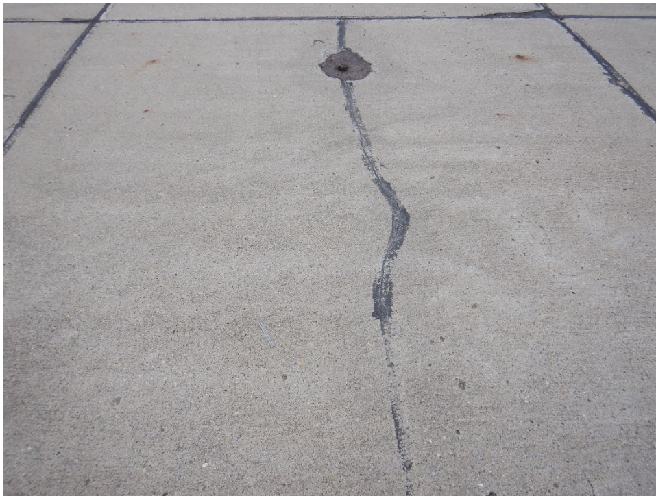
A01LE-02. LTD Cracking (Sample Unit No. 05).
