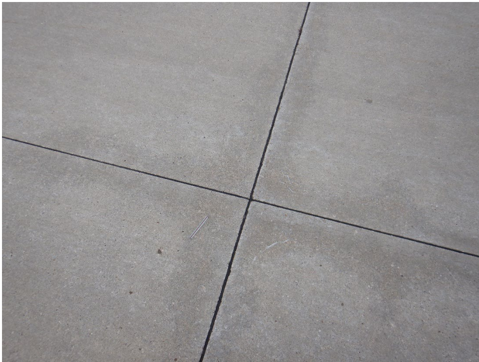
R18LE-05. Durability Cracking (Sample Unit No. 02).
