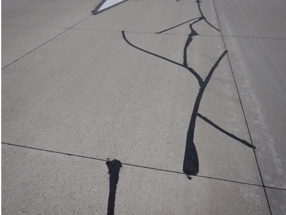
R18LE-05. Shattered Slab (Sample Unit No. 05) (1).
