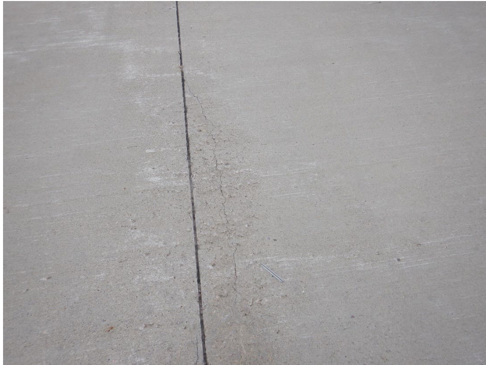
R18LE-07. Joint Spalling (Sample Unit No. 08).
