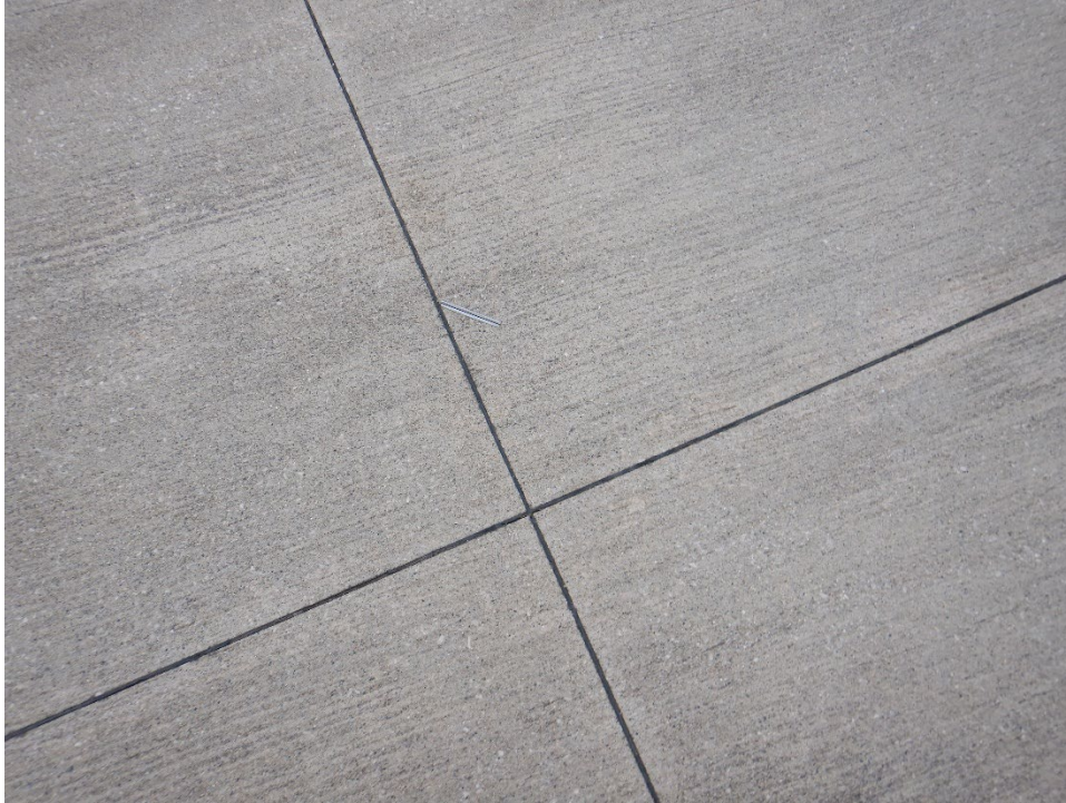
R18LE-04. Joint Seal Damage (Sample Unit No. 01).
