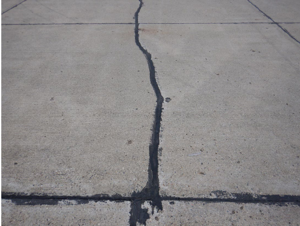
A01LE-01. LTD Cracking (Sample Unit No. 03).
