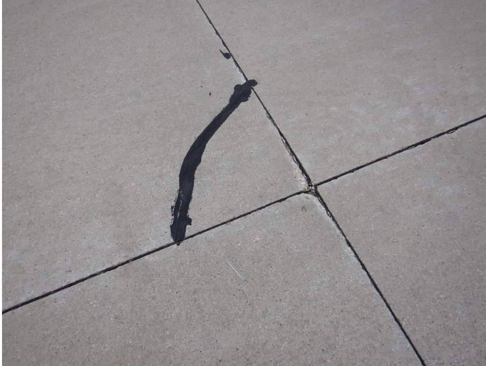
R18LE-05. Corner Break (Sample Unit No. 05).
