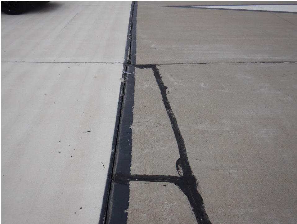
R18LE-07. Faulting (Additional Sample Unit No. 01).
