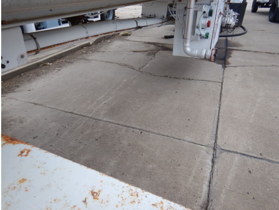
A01LE-02. Shattered Slab (Sample Unit No. 04).
