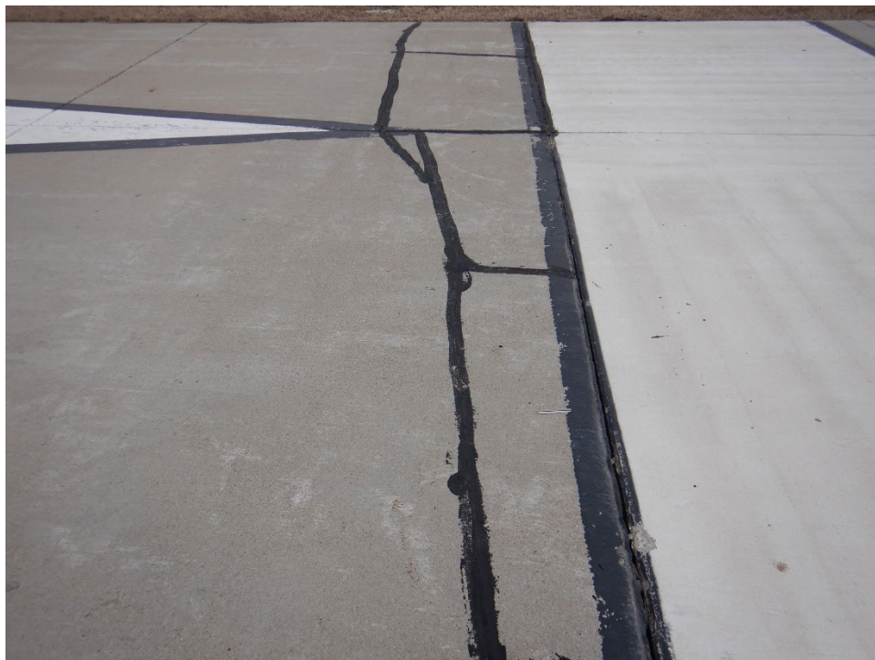
R18LE-07. LTD Cracking (Additional Sample Unit No. 01).
