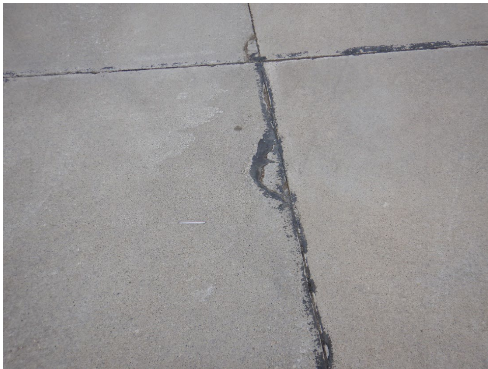
TH01LE-01. Joint Spalling (Sample Unit No. 01).
