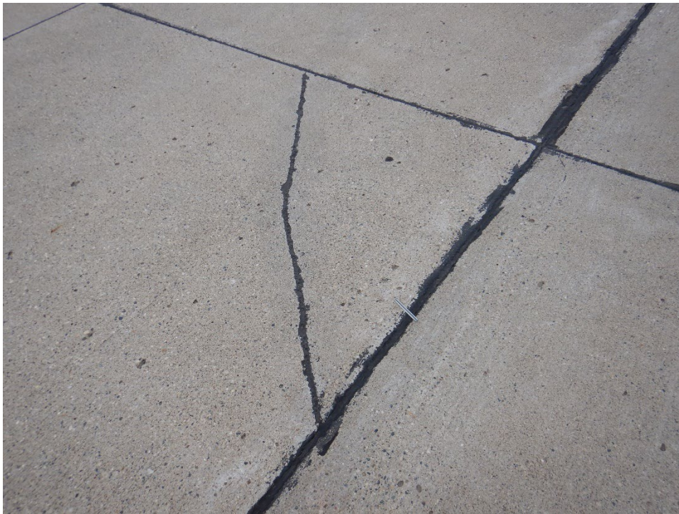
A01LE-01. Corner Break (Sample Unit No. 03).
