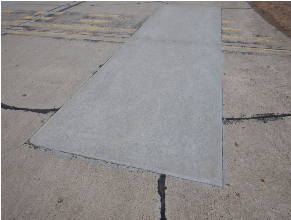
T01LE-01. Large Patching (Sample Unit No. 01).
