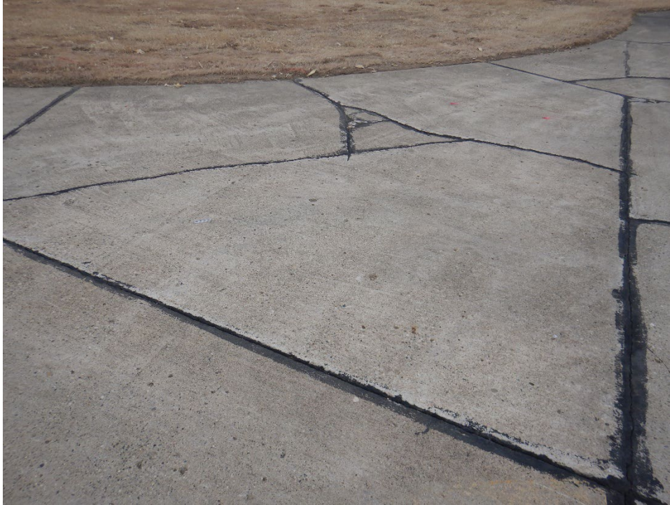
T01LE-01. Shattered Slab (Sample Unit No. 01).
