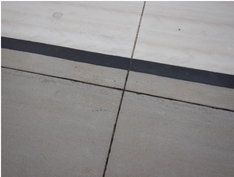
R18LE-06. Joint Seal Damage (Sample Unit No. 03).
