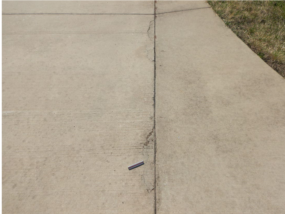
TH01LA-02. Joint Spalling (Sample Unit No. 01).
