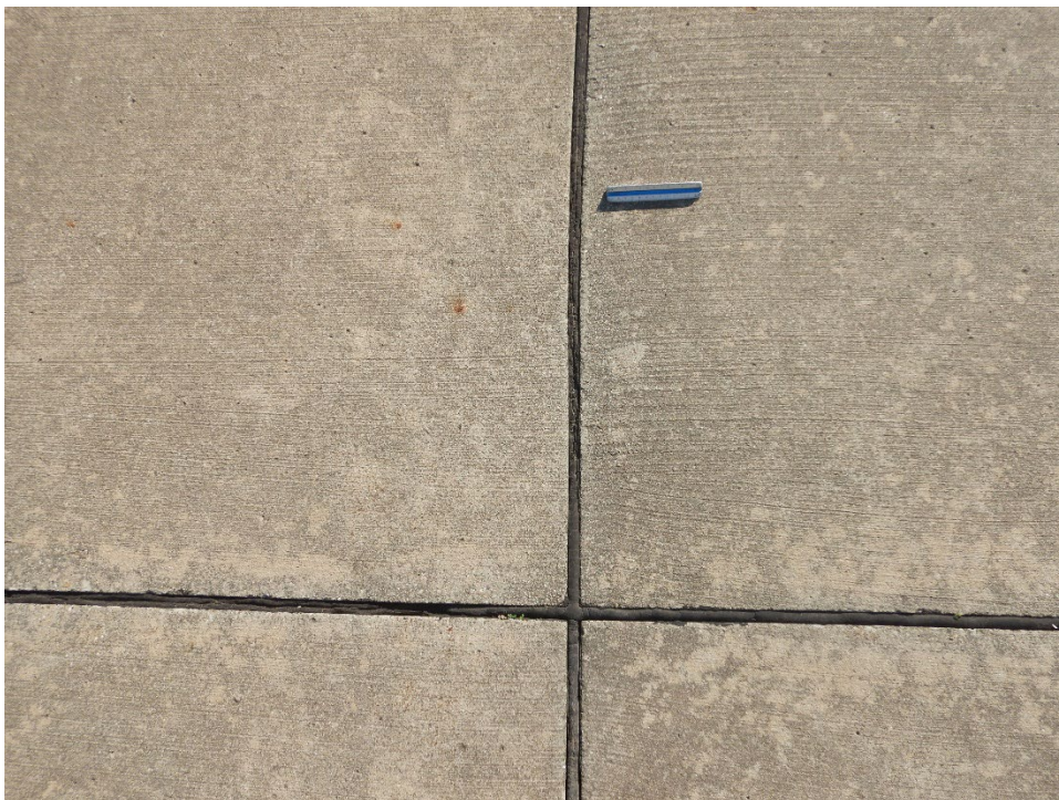
T02LA-01. Joint Seal Damage (Sample Unit No. 01).
