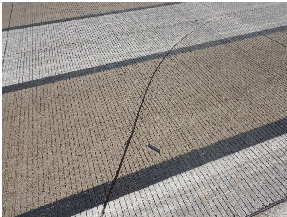
R18LA-01. LTD Cracking (Sample Unit No. 05).
