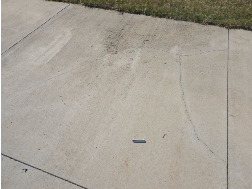
R18LA-02. Shattered Slab (Sample Unit No. 13).
