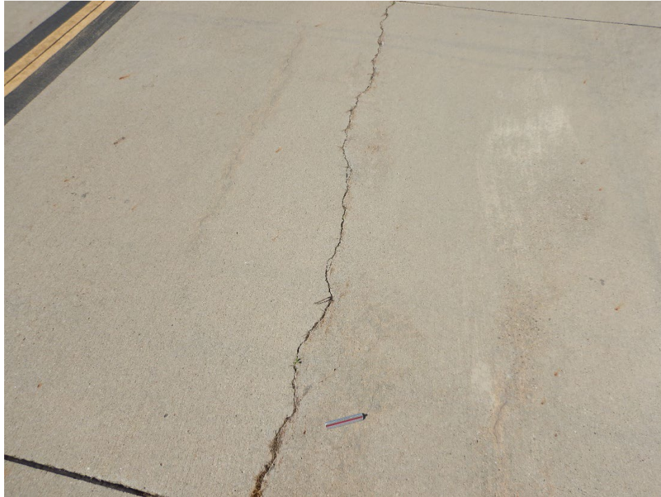
TH01LA-01. LTD Cracking (Additional Sample Unit No. 07).
