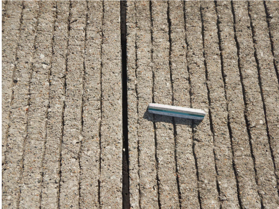
R18LA-01. Joint Seal Damage (Sample Unit No. 05).
