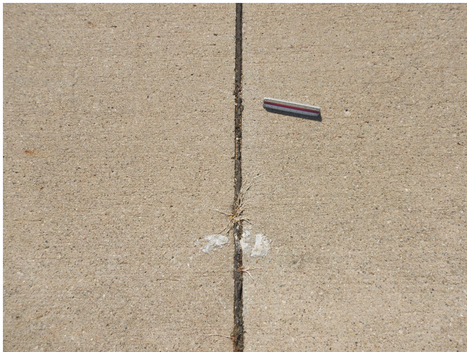
T01LA-01. Joint Seal Damage (Sample Unit No. 02).
