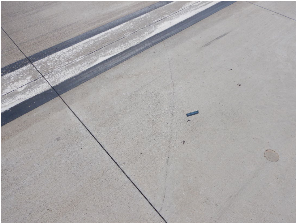
R18LA-02. LTD Cracking (Sample Unit No. 03).
