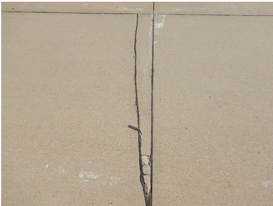
A01LA-01. Joint Spalling (Sample Unit No. 02).
