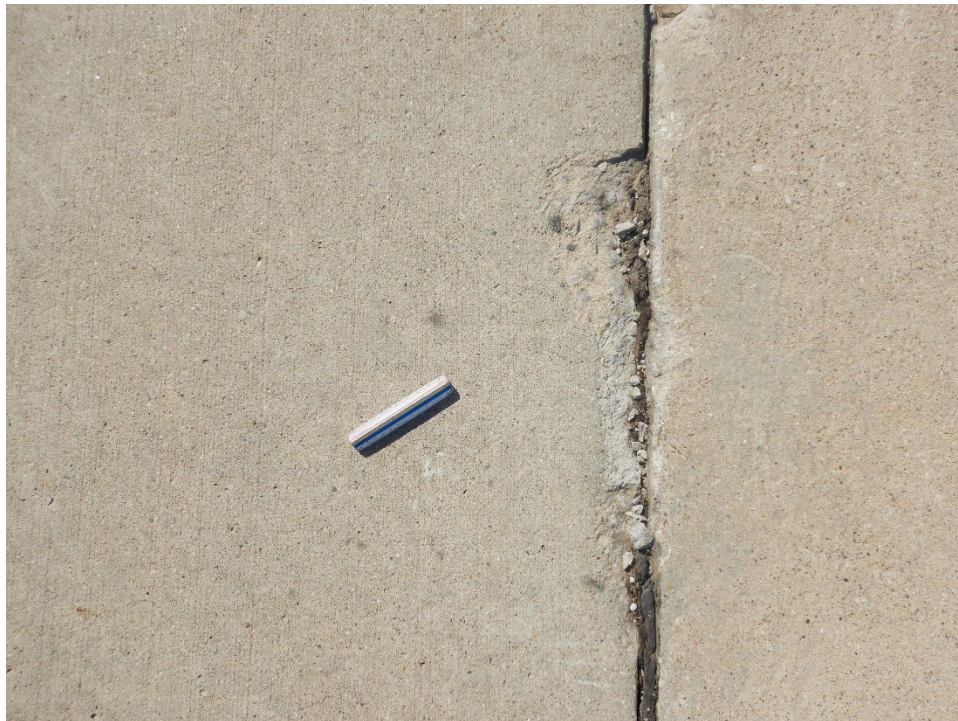
TH01LA-01. Joint Spalling (Sample Unit No. 01).
