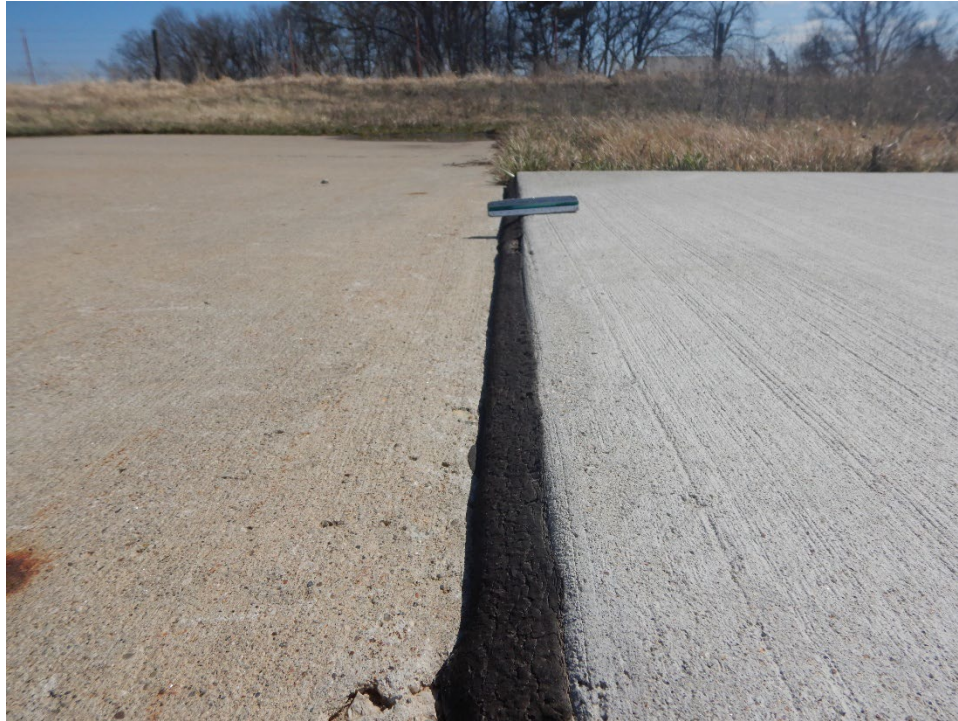
TH01LA-01. Faulting (Sample Unit No. 10).
