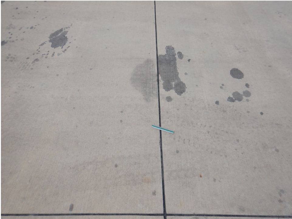
TH01LA-02. Joint Seal Damage (Sample Unit No. 02).
