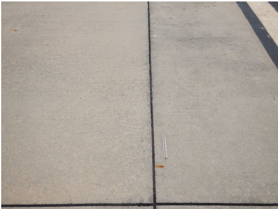
T02LA-01. Joint Seal Damage (Sample Unit No. 04).
