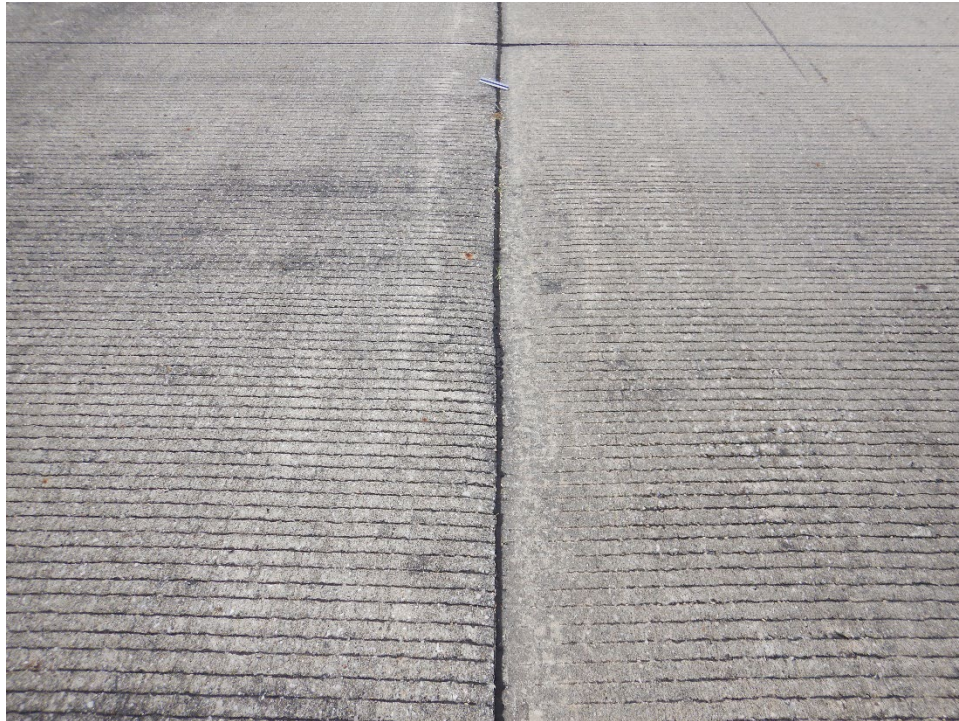
R18LA-01. Joint Seal Damage (Sample Unit No. 14).
