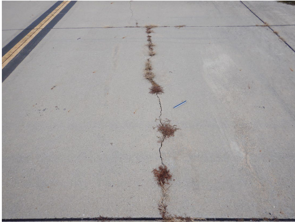
TH01LA-01. LTD Cracking (Additional Sample Unit No. 07).
