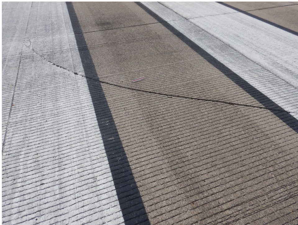
R18LA-01. LTD Cracking (Sample Unit No. 05).
