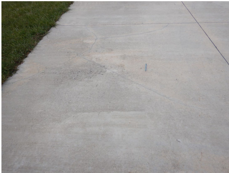
R18LA-02. Shattered Slab (Sample Unit No. 13).
