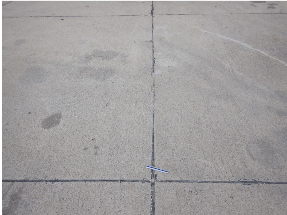
A01LA-01. Joint Seal Damage (Sample Unit No. 05).
