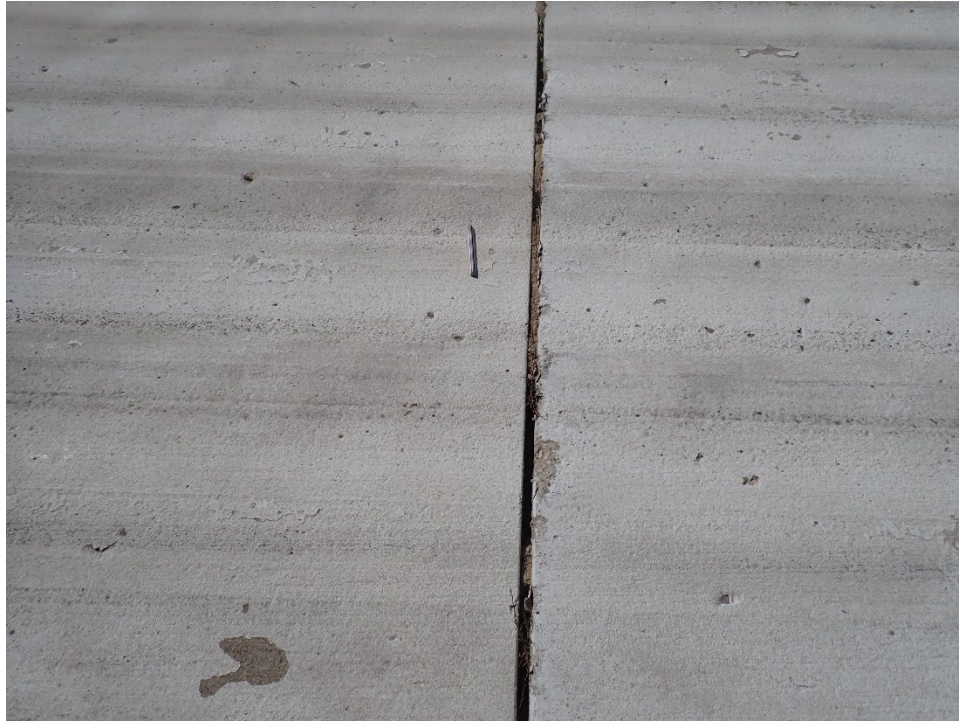
R15KN-02. Joint Seal Damage (Sample Unit No. 16).
