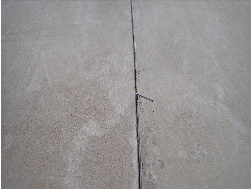
TBKN-05. Joint Seal Damage (Sample Unit No. 04).
