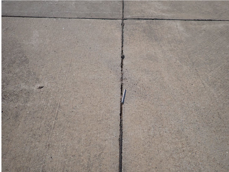
TCKN-01. Joint Seal Damage (Sample Unit No. 02).
