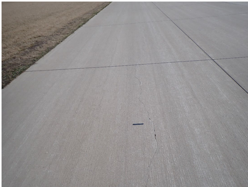
R15KN-01. LTD Cracking (Sample Unit No. 07).
