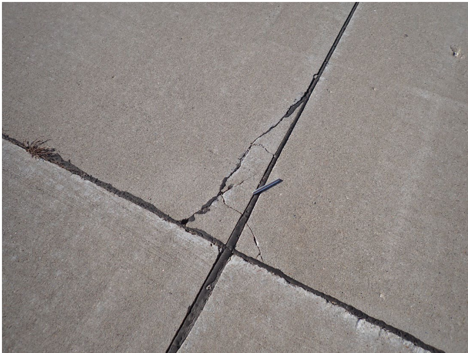
A02KN-01. Joint Spalling (Sample Unit No. 10).
