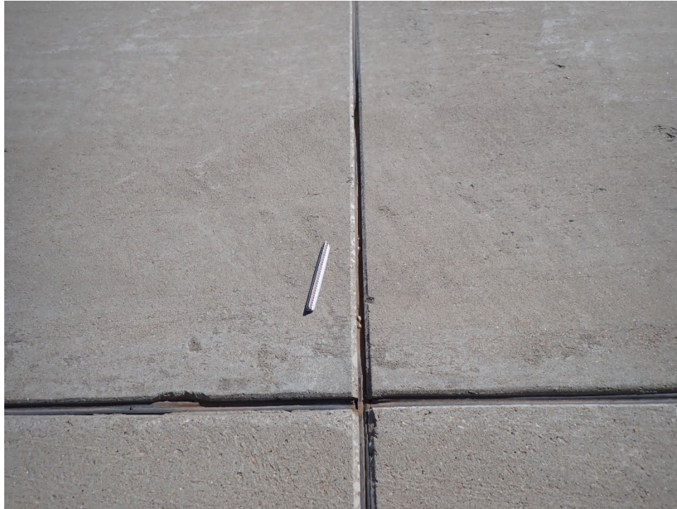
R15KN-01. Joint Seal Damage (Sample Unit No. 57).
