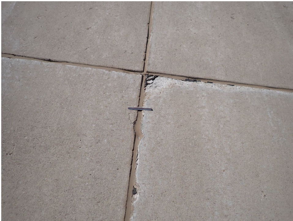
TBKN-03. Faulting (Sample Unit No. 05).
