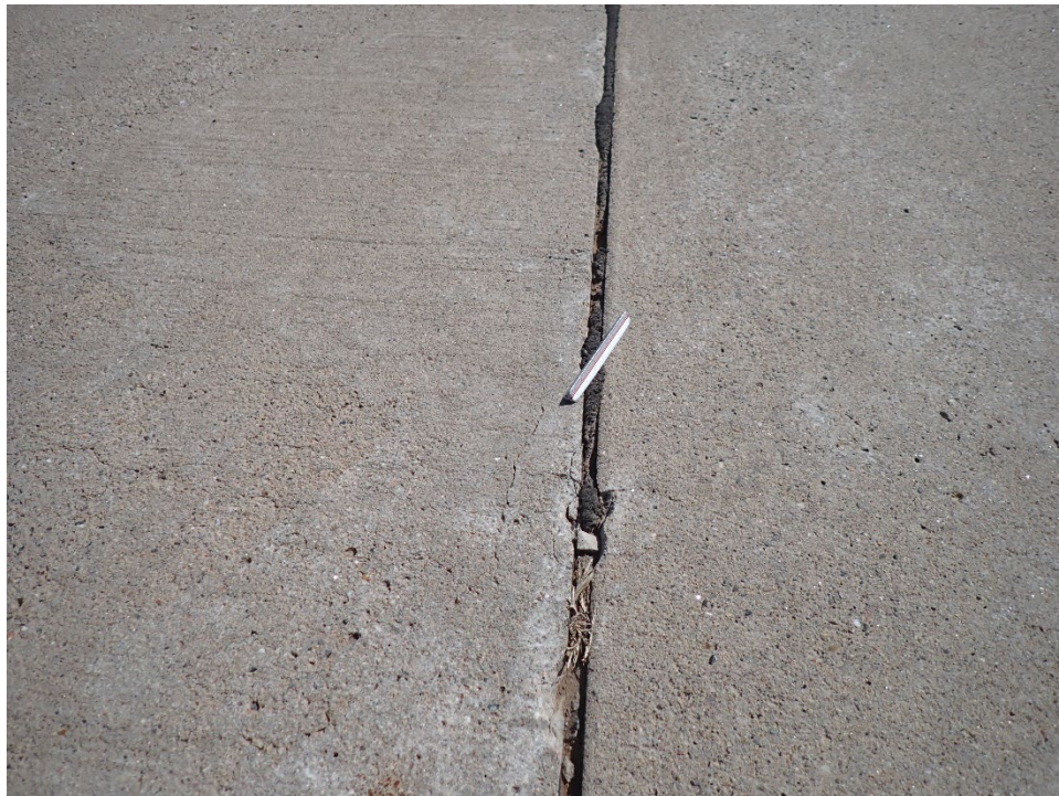
TBKN-04. Joint Spalling (Sample Unit No. 01).
