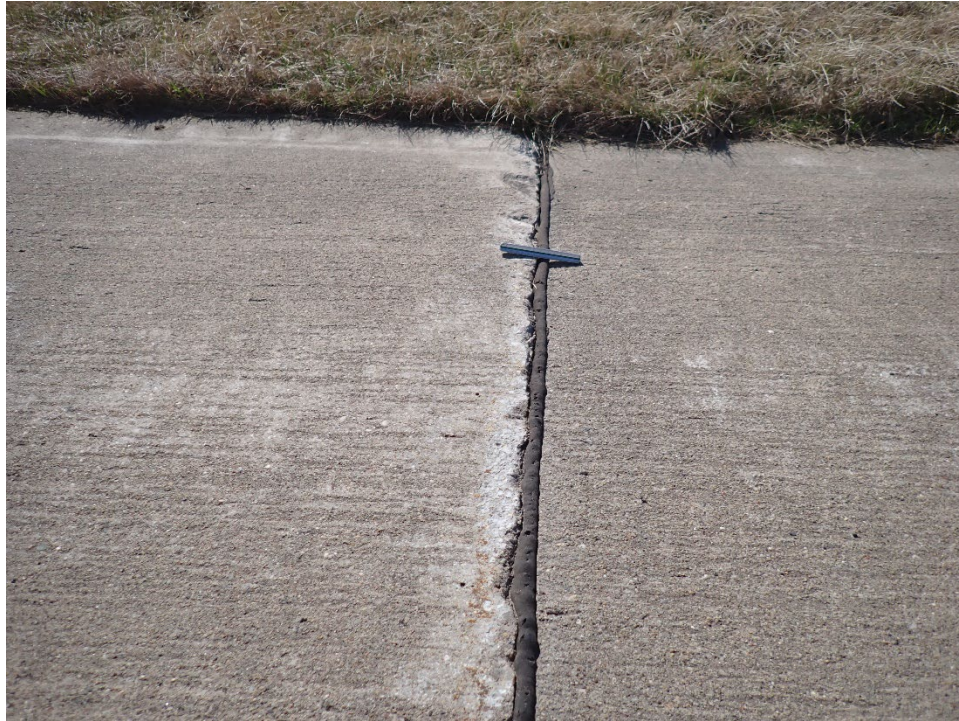
TBKN-02. Faulting (Sample Unit No. 20).
