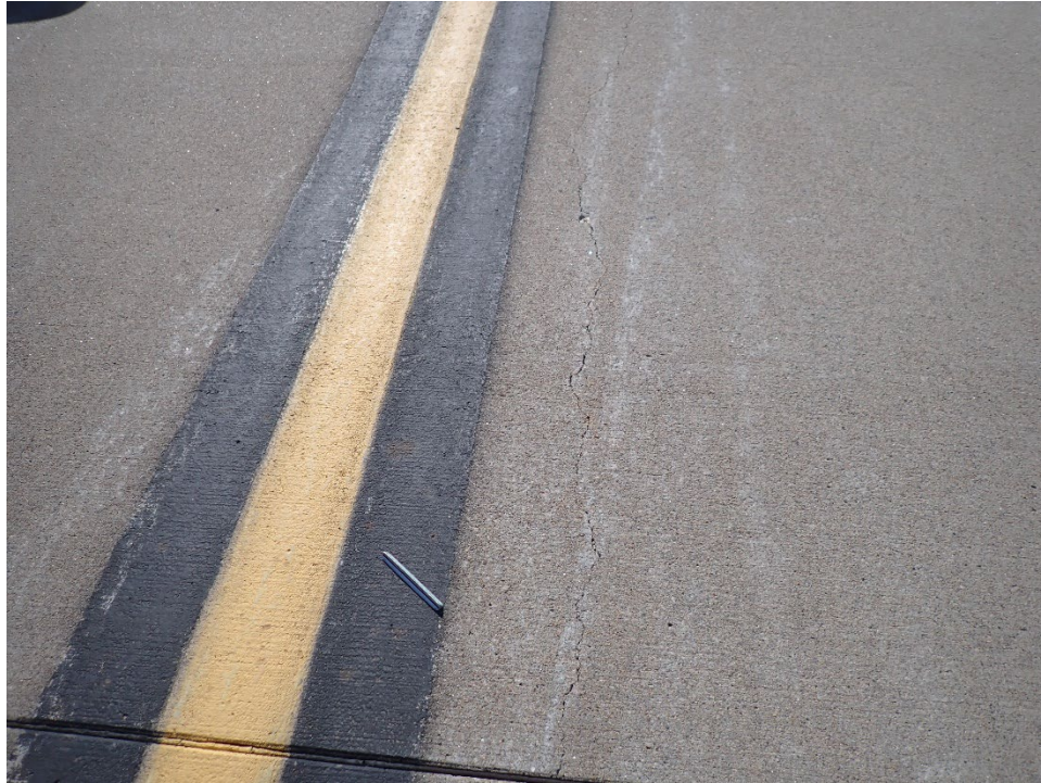
TAKN-01. Shrinkage Cracking (Sample Unit No. 04).
