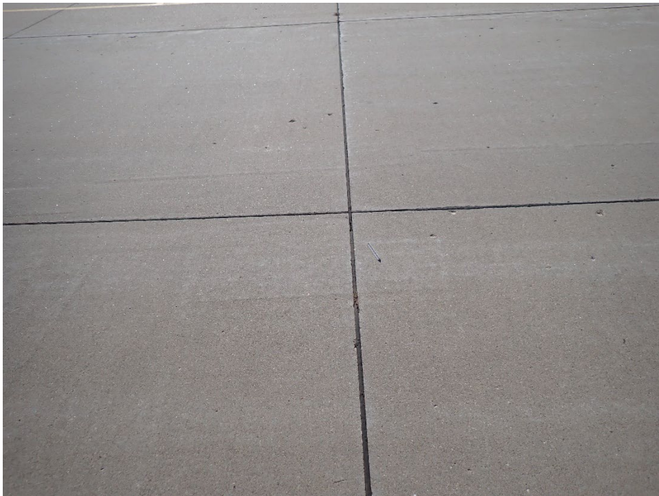
A02KN-01. Joint Seal Damage (Sample Unit No. 08).
