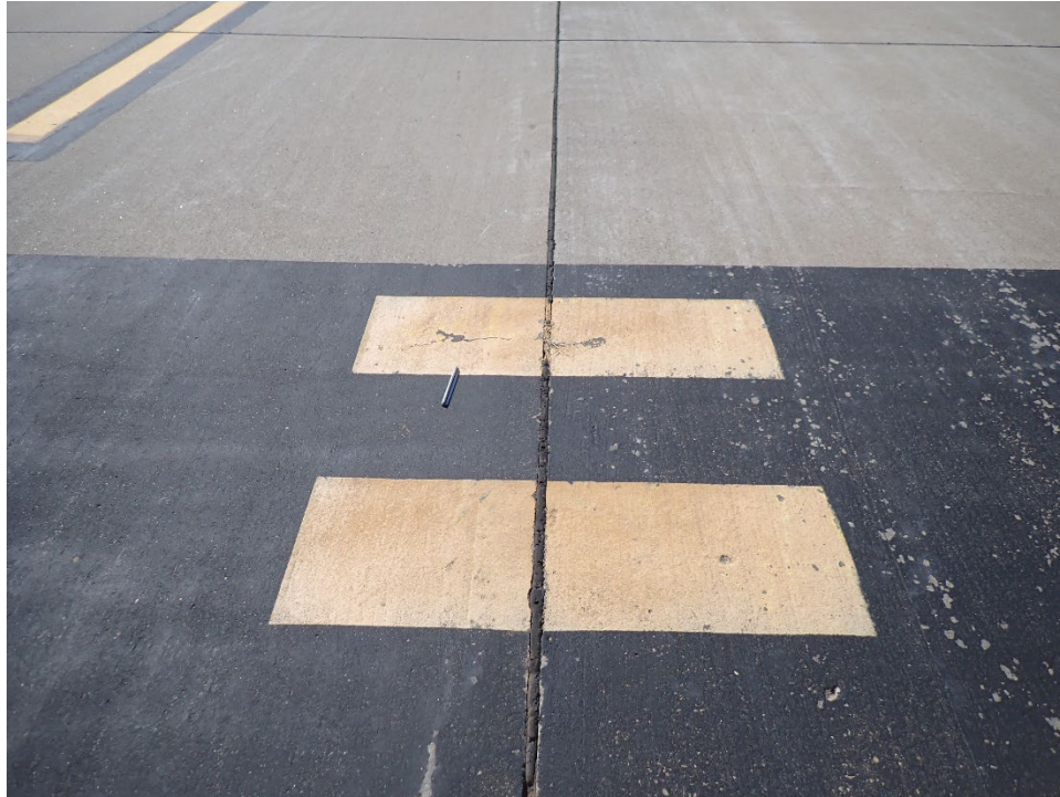
TBKN-04. Joint Seal Damage (Sample Unit No. 01).
