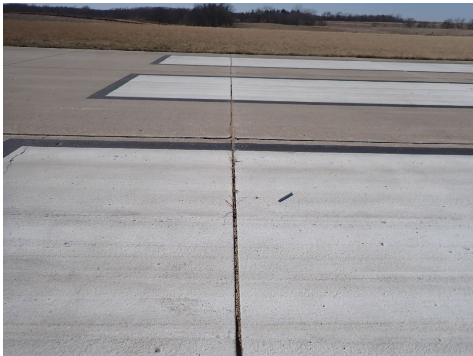
R15KN-02. Joint Seal Damage (Sample Unit No. 19) (1).
