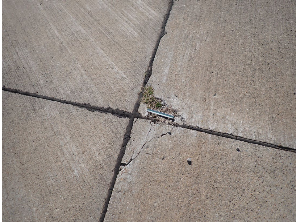
TCKN-01. Corner Spalling (Sample Unit No. 02) (1).
