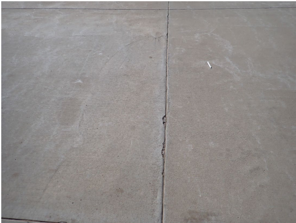
A01KN-01. Joint Seal Damage (Sample Unit No. 02).
