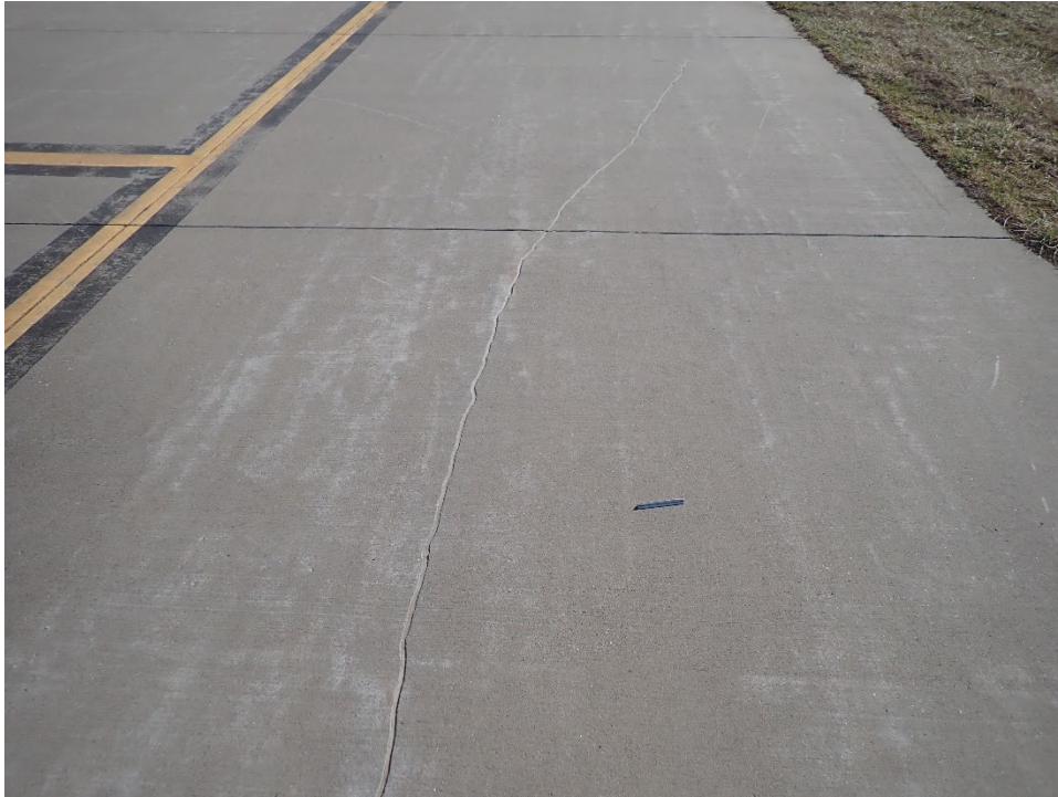
TH01KN-02. LTD Cracking (Sample Unit No. 02).
