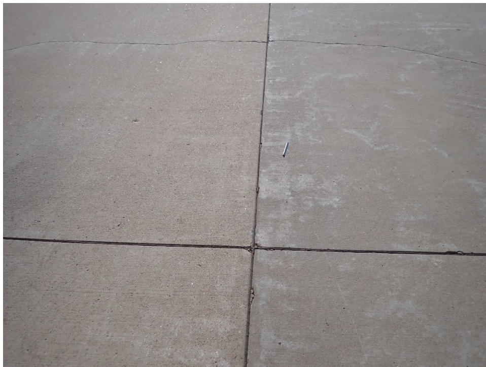
A02KN-02. Joint Seal Damage (Sample Unit No. 03).
