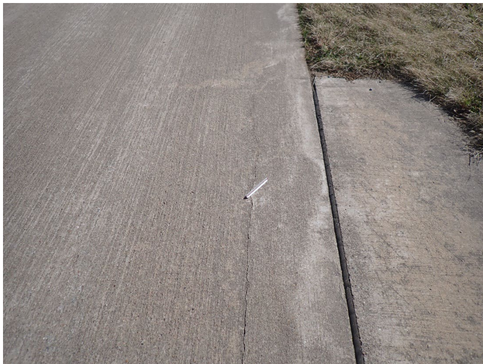
TBKN-02. Shrinkage Cracking (Sample Unit No. 23).
