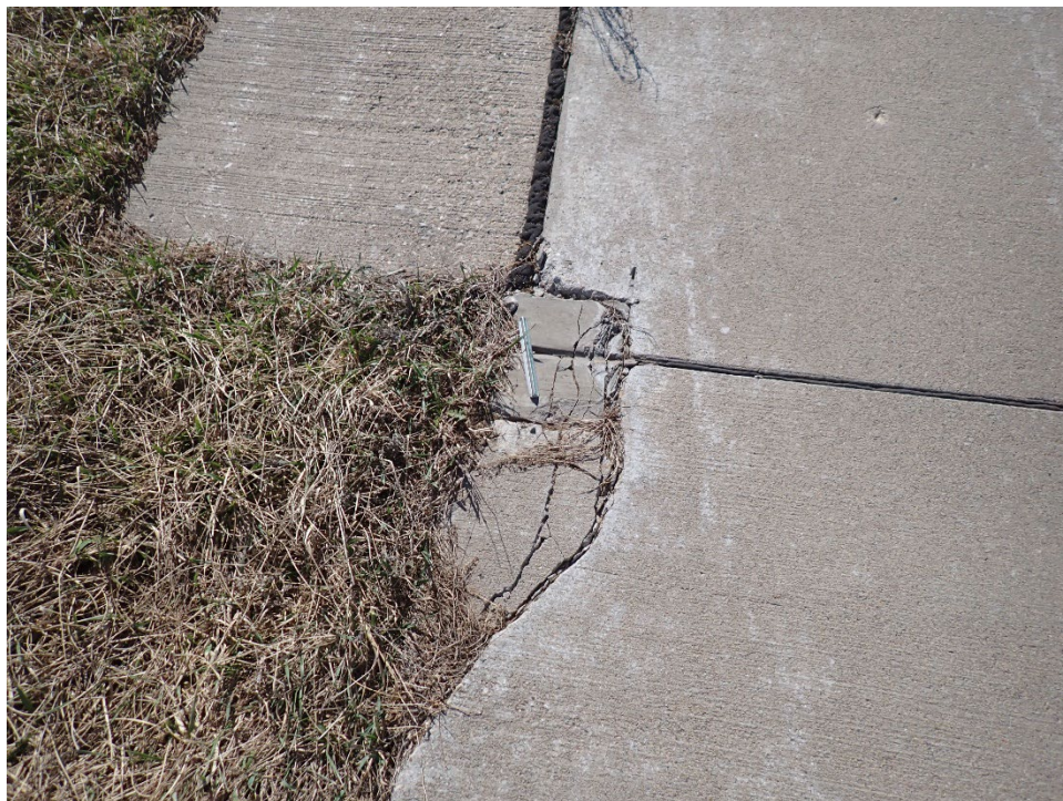
TAKN-01. Small Patching (Sample Unit No. 04).
