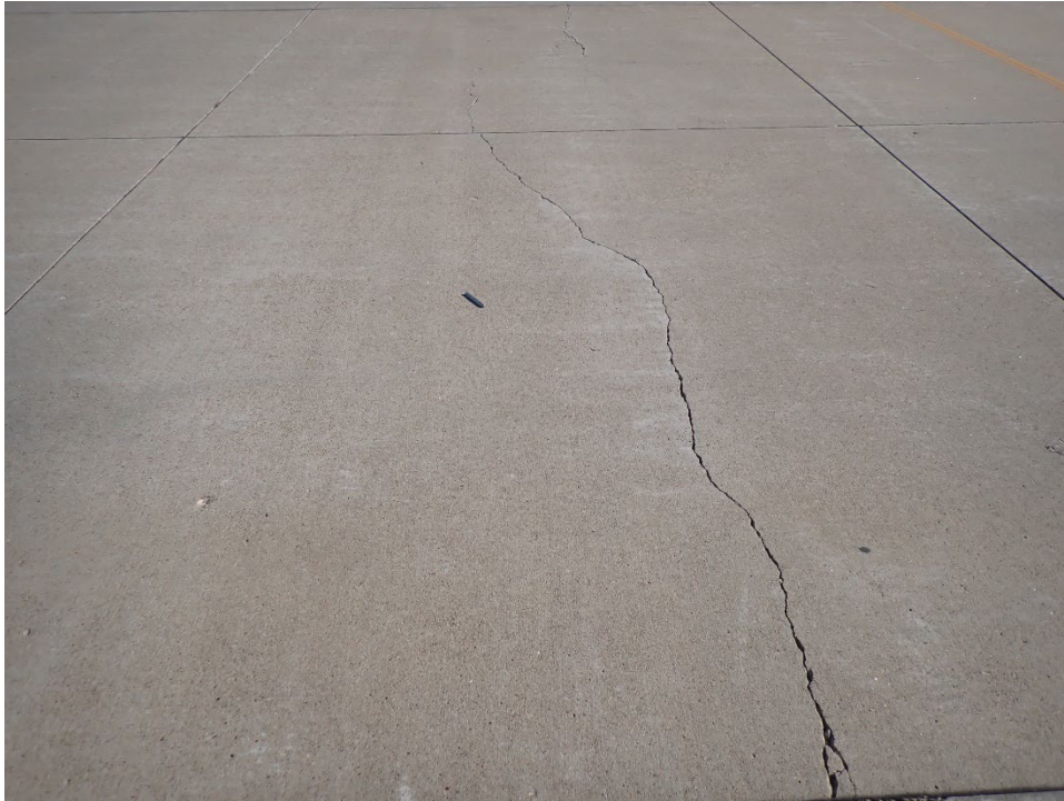
A02KN-02. LTD Cracking (Sample Unit No. 03).
