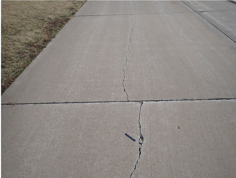
TBKN-01. LTD Cracking (Sample Unit No. 12).
