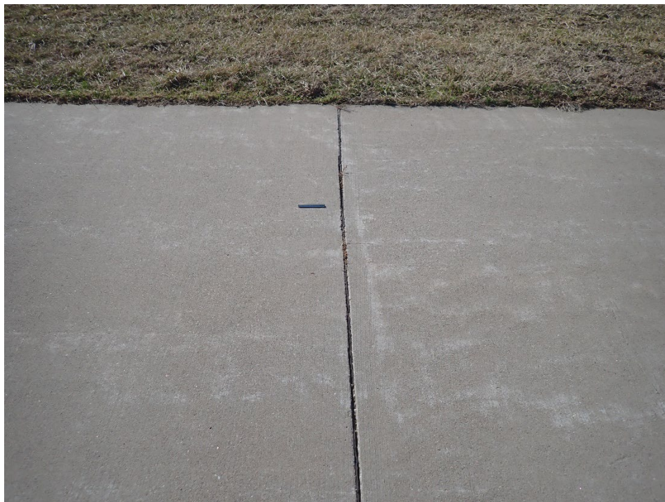
TH01KN-02. Joint Seal Damage (Sample Unit No. 01).
