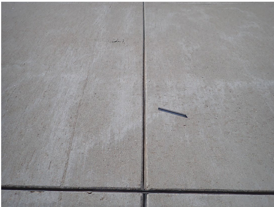
TBKN-05. Joint Seal Damage (Sample Unit No. 01).
