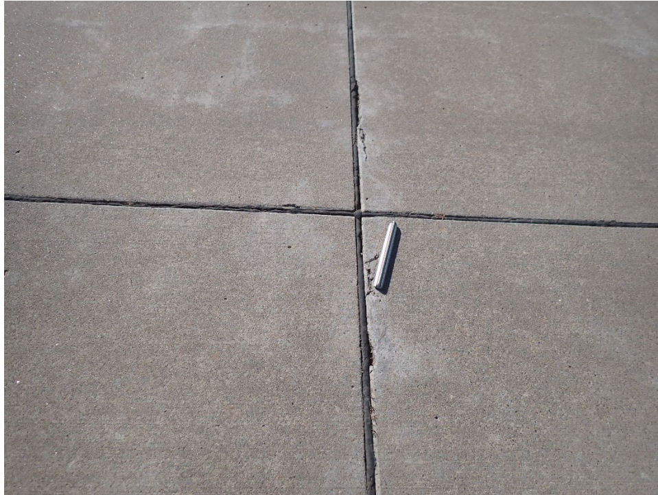
A01KN-01. Joint Spalling (Sample Unit No. 04).
