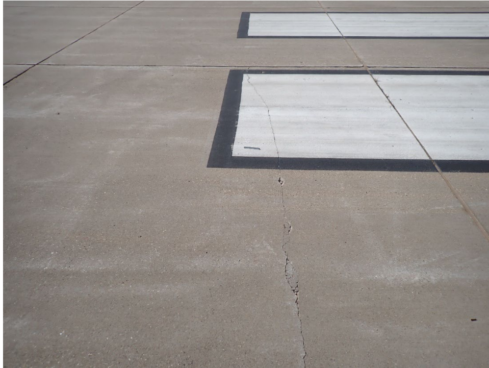
R15KN-02. LTD Cracking (Sample Unit No. 19).
