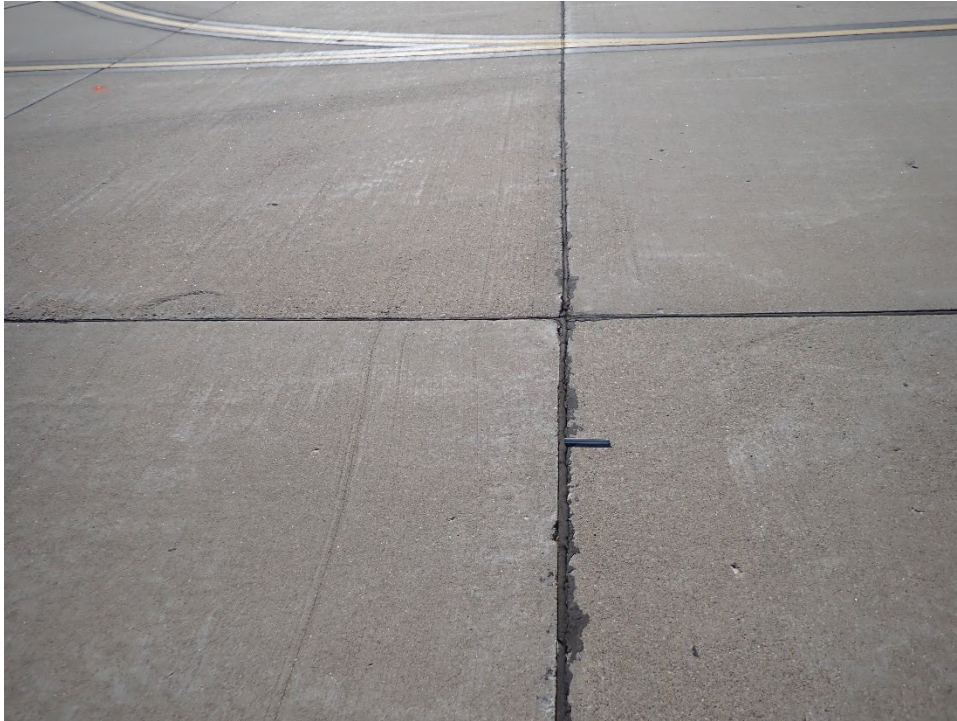
A02KN-01. Joint Seal Damage (Sample Unit No. 10).
