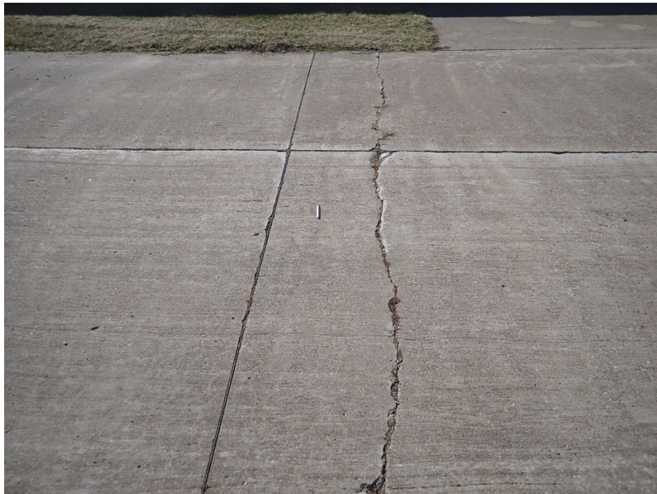
TH01KN-01. LTD Cracking (Sample Unit No. 04).
