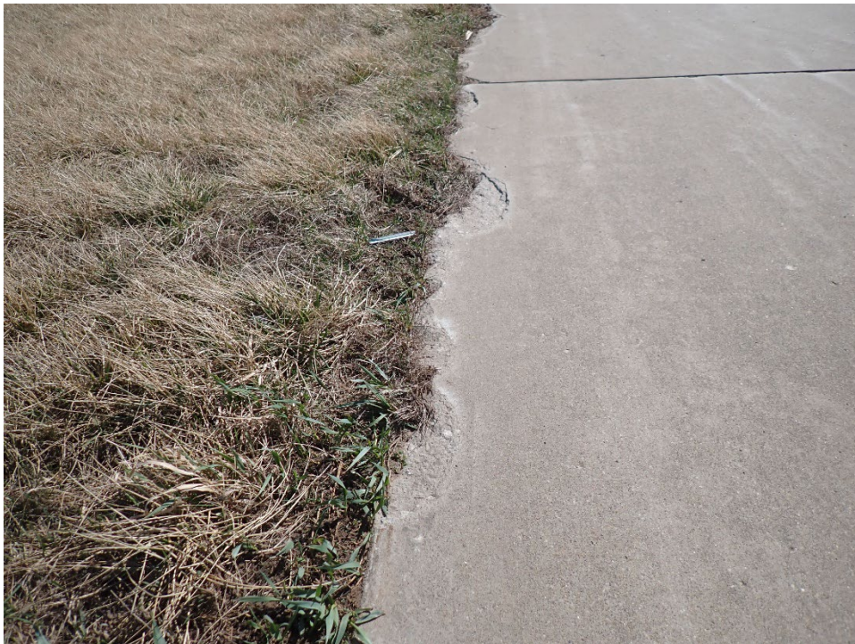
R15KN-02. Joint Spalling (Sample Unit No. 02).
