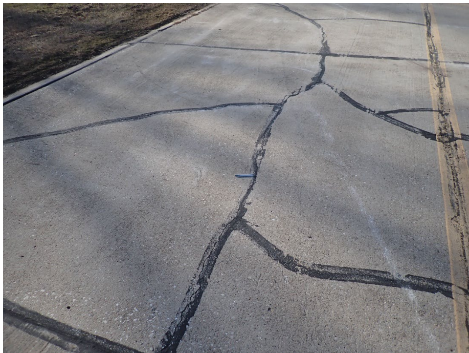
A01JE-03. Shattered Slab (Sample Unit No. 03).
