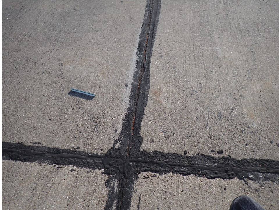
A01JE-03. Joint Seal Damage (Sample Unit No. 01).
