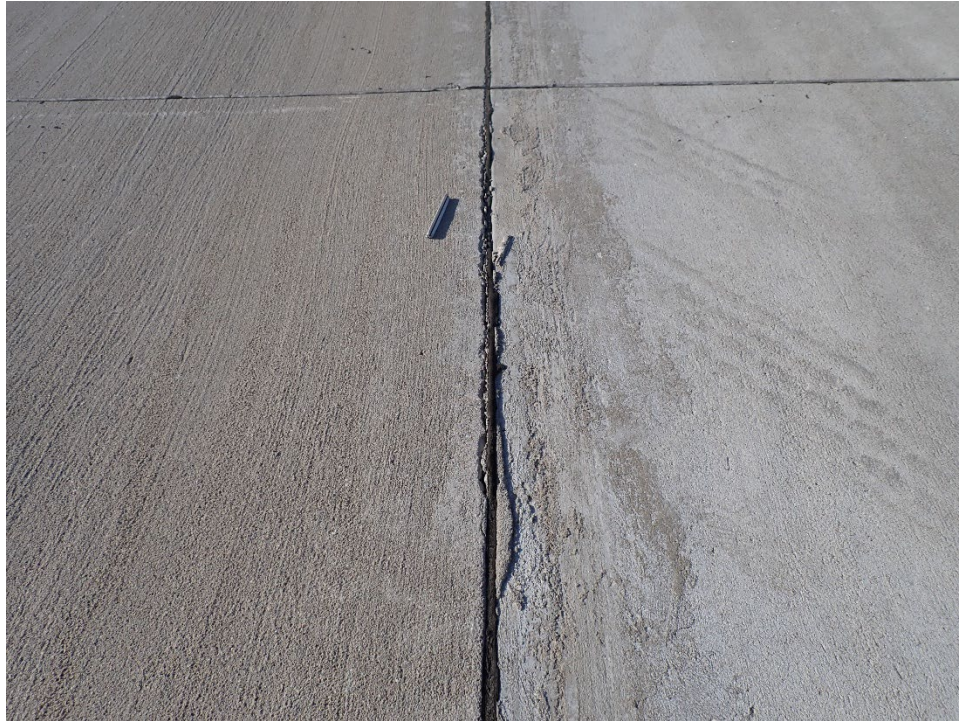
R14JE-04. Joint Seal Damage (Sample Unit No. 10).
