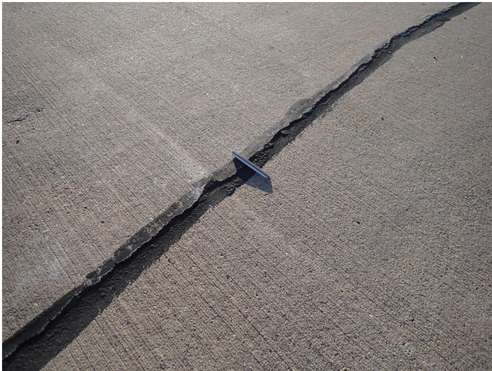
A02JE-01. Faulting (Sample Unit No. 05).
