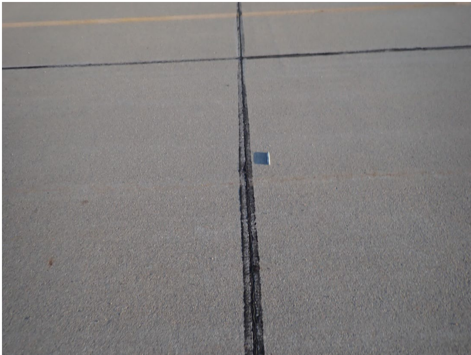
A01JE-02. Joint Seal Damage (Sample Unit No. 01).
