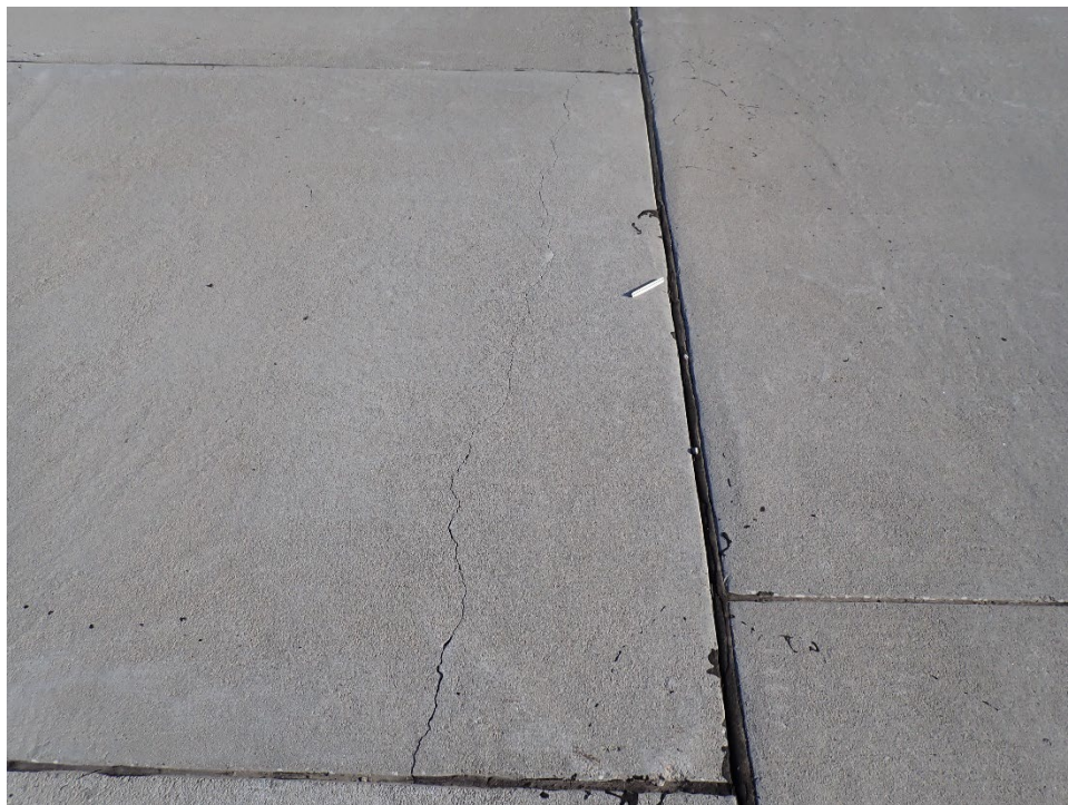
R14JE-04. LTD Cracking (Sample Unit No. 19).
