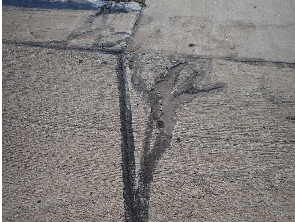
A01JE-01. Joint Spalling (Additional Sample Unit No. 12).
