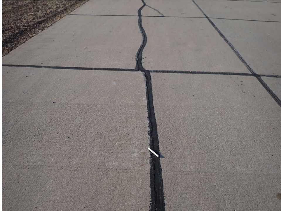
A02JE-01. LTD Cracking (Sample Unit No. 07).
