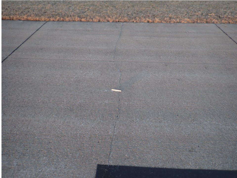
R14JE-01. LTD Cracking (Sample Unit No. 05).
