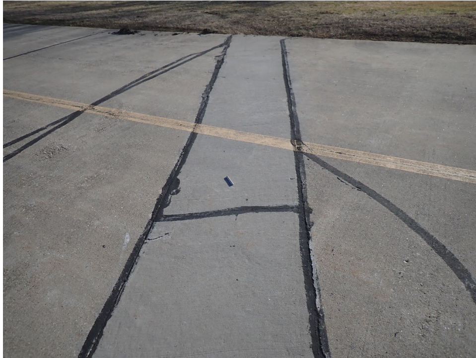
A01JE-01. Large Patching (Sample Unit No. 03).
