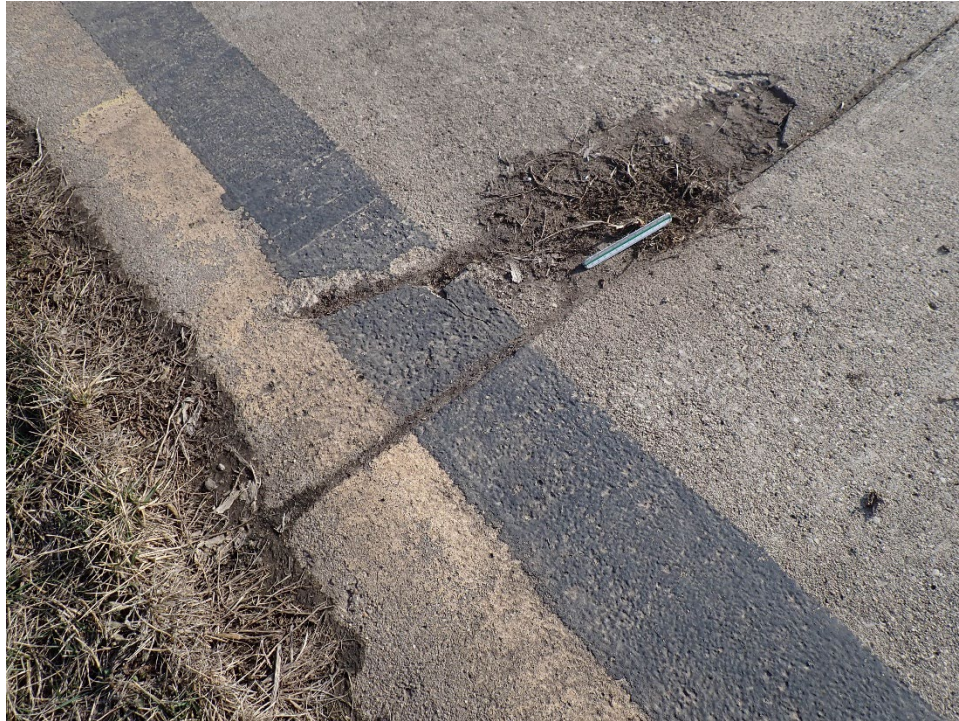
R14JE-03. Joint Spalling (Sample Unit No. 05).
