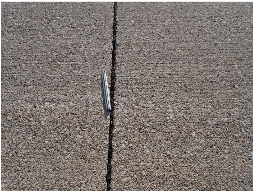
R14JE-03. Joint Seal Damage (Sample Unit No. 02).
