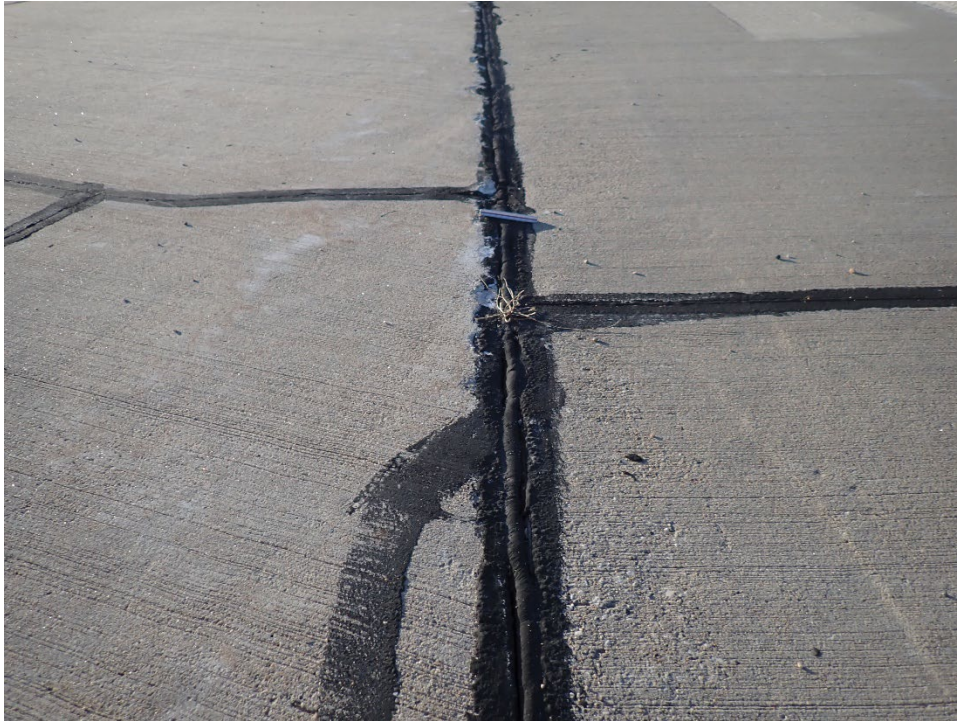
A02JE-02. Faulting (Sample Unit No. 02).
