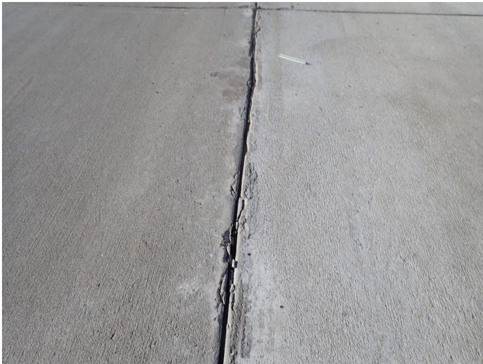
R14JE-04. Joint Seal Damage (Sample Unit No. 04).
