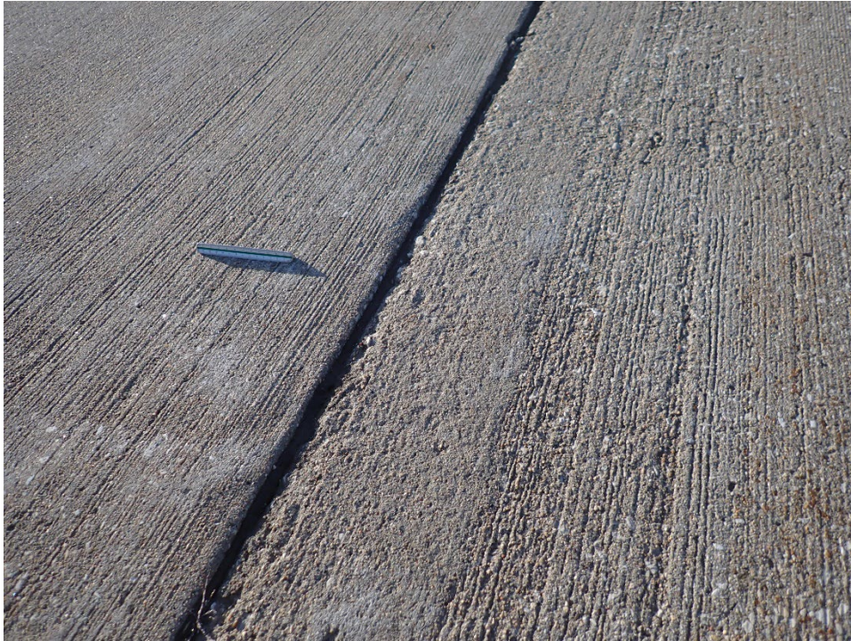
A01JE-01. Joint Seal Damage (Sample Unit No. 15) (1).
