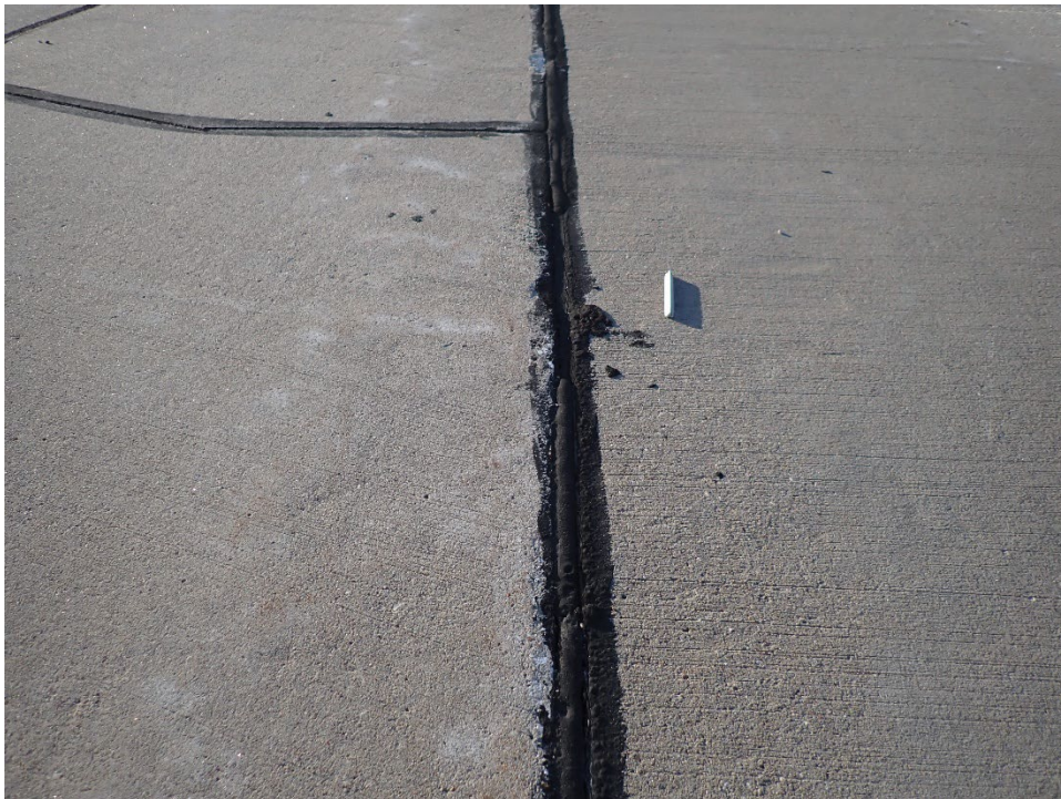
A02JE-02. Joint Seal Damage (Sample Unit No. 02).
