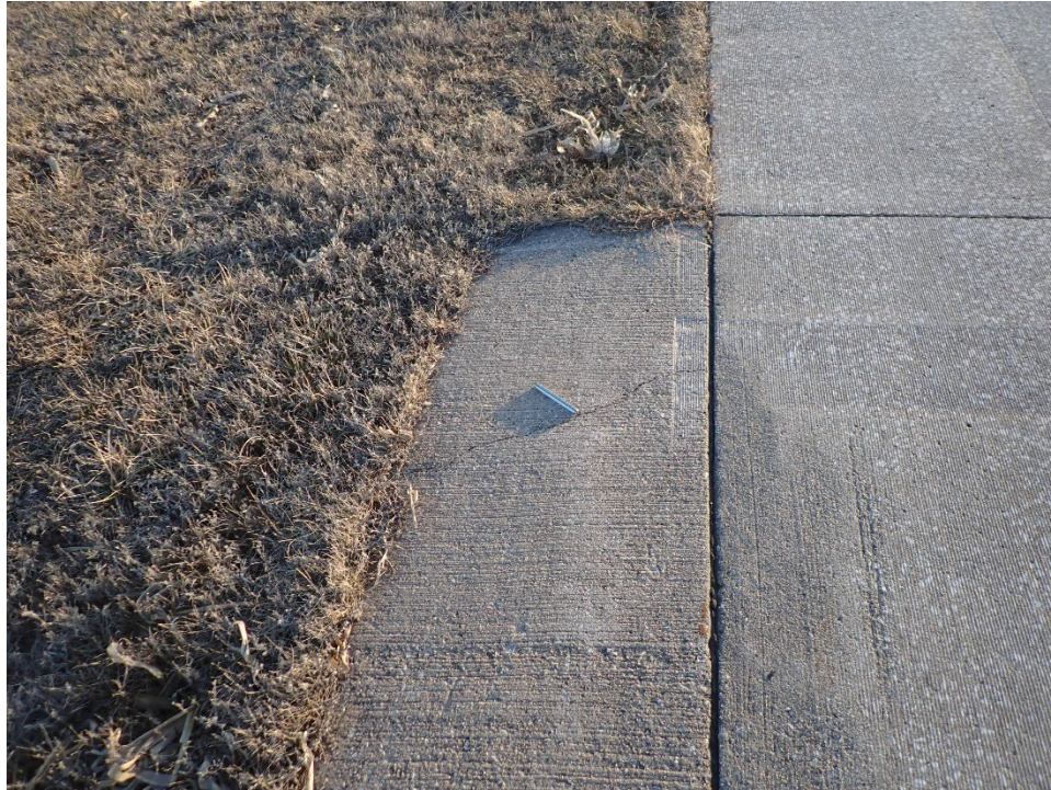
T01JE-01. LTD Cracking (Sample Unit No. 05).
