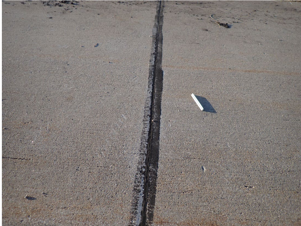
T02JE-01. Joint Seal Damage (Sample Unit No. 01).
