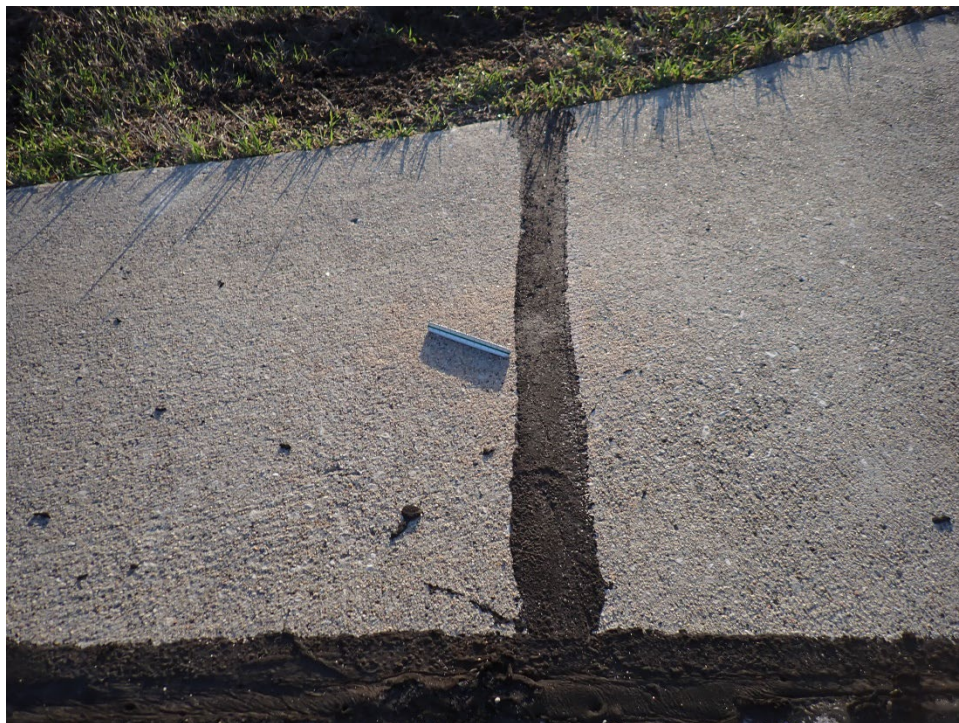
T02JE-01. LTD Cracking (Sample Unit No. 03).
