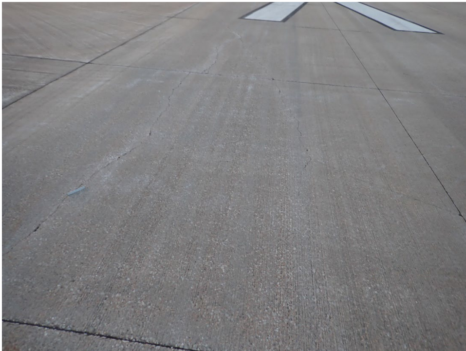
R14JE-02. Shattered Slab (Sample Unit No. 04).
