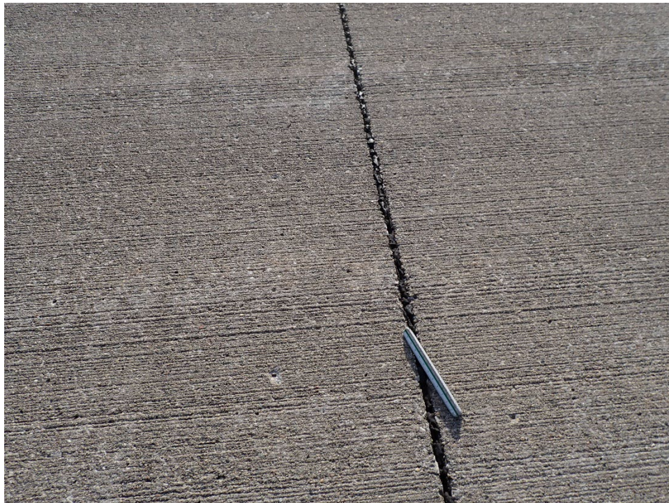
R14JE-01. Joint Seal Damage (Sample Unit No. 44).
