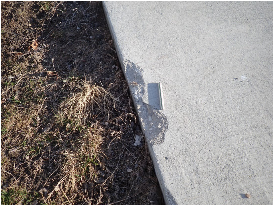
A02JE-03. Joint Spalling (Sample Unit No. 04).
