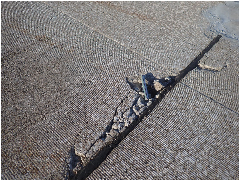
A01JE-01. Joint Spalling (Additional Sample Unit No. 18).
