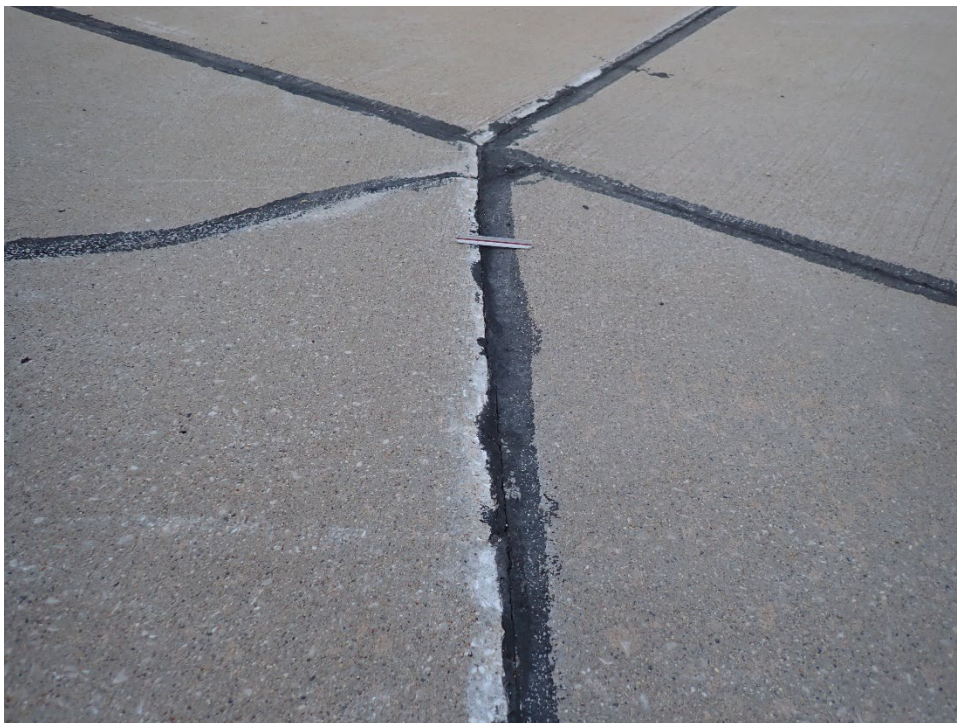
A01JE-01. Faulting (Sample Unit No. 20).
