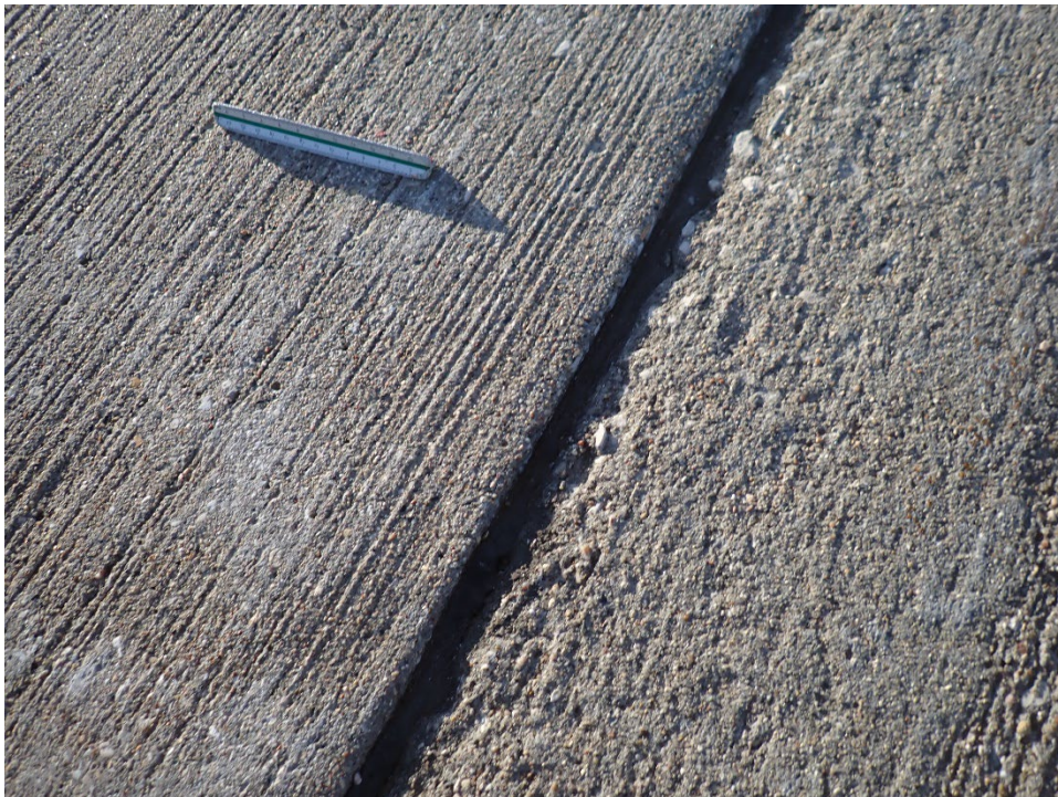
A01JE-01. Joint Seal Damage (Sample Unit No. 15) (2).
