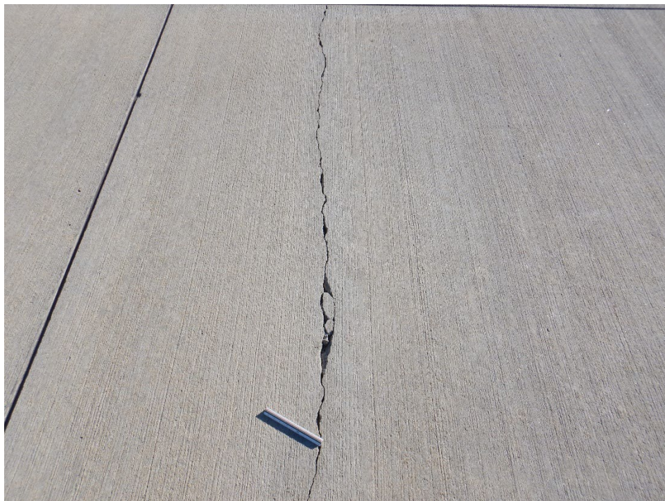
TAIC-02. LTD Cracking (Additional Sample Unit No. 089).
