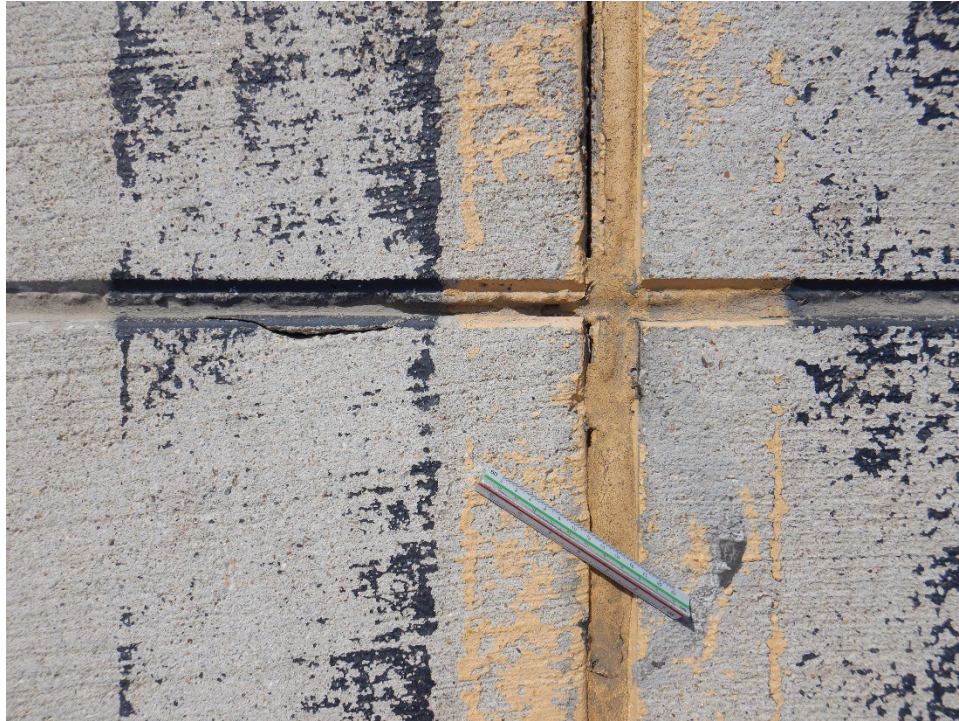
TBIC-02. Joint Seal Damage (Sample Unit No. 01).
