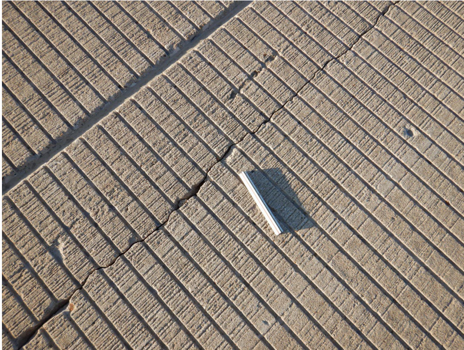
R07IC-03. LTD Cracking (Sample Unit No. 16) (4).
