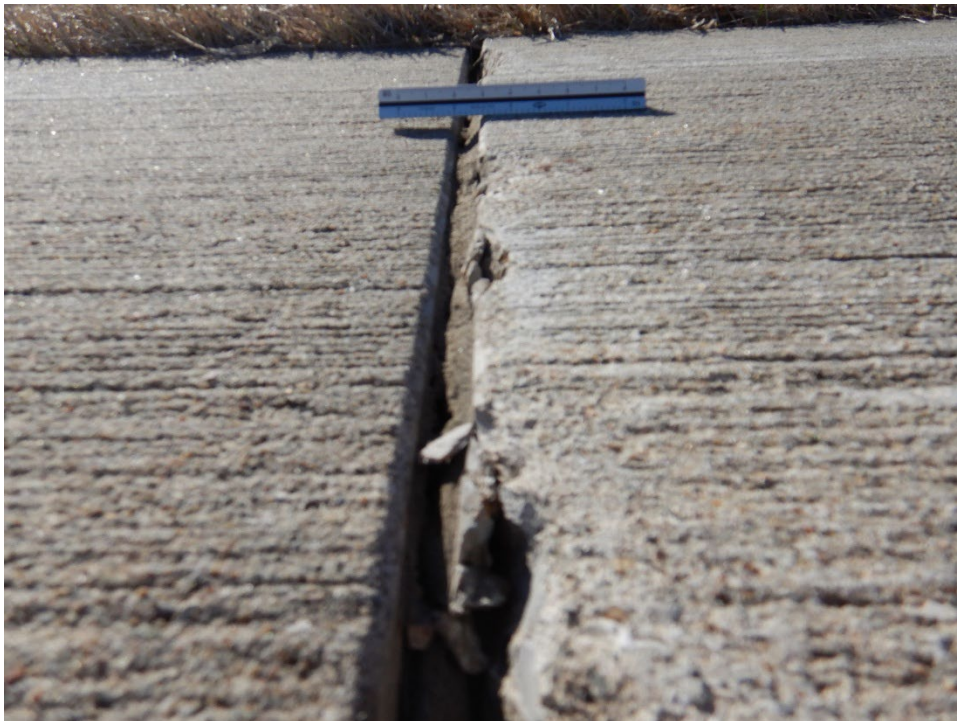
TAIC-02. Faulting (Sample Unit No. 015).
