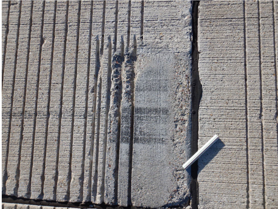
R07IC-01 Small Patching. (Additional Sample Unit No. 36) (3).
