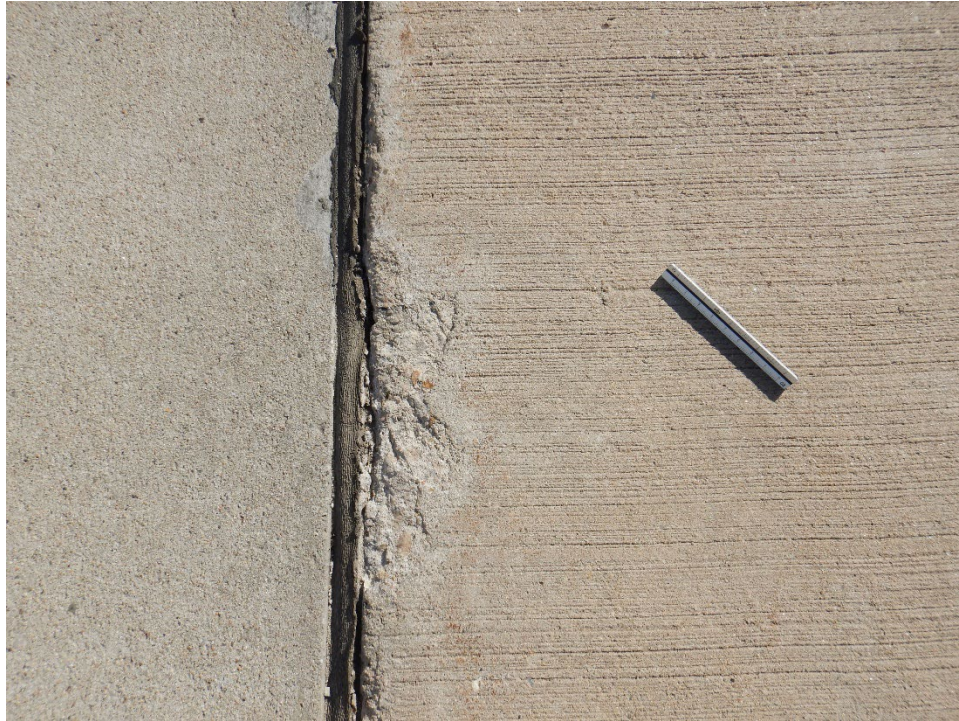
TH02IC-05. Joint Spalling (Sample Unit No. 01).
