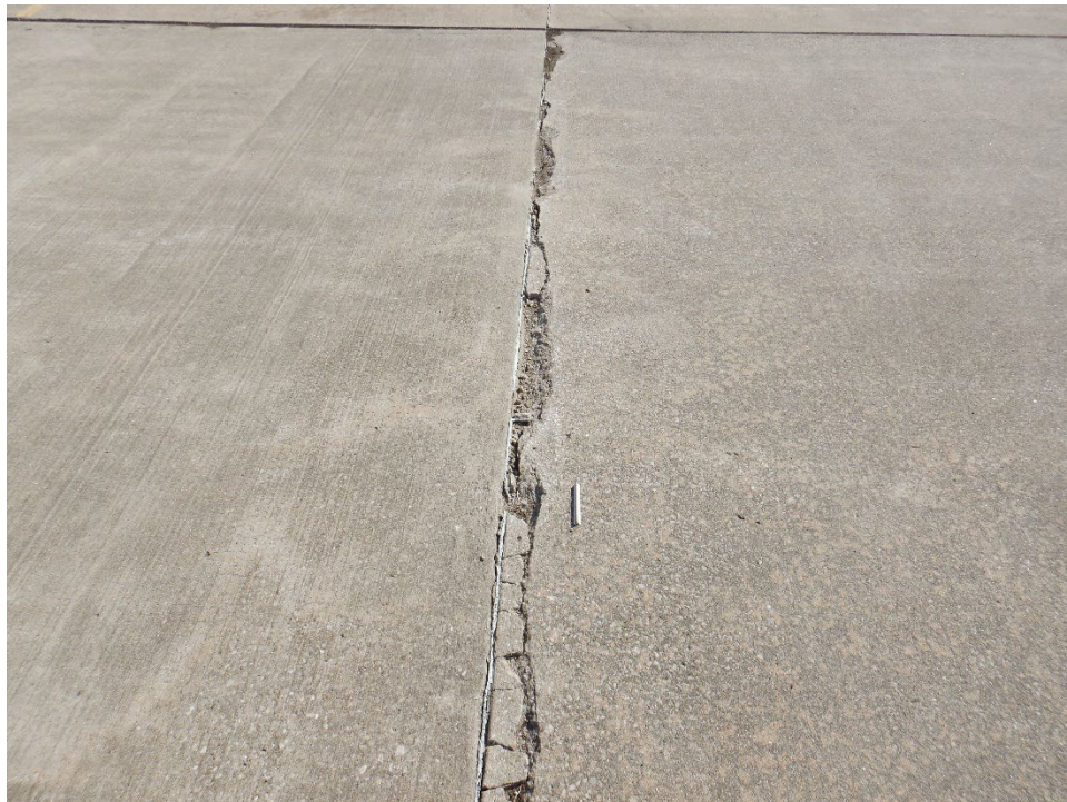
TH02IC-02. Joint Spalling (Sample Unit No. 13).
