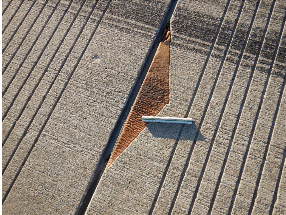
R07IC-02 Small Patching. (Sample Unit No. 08).
