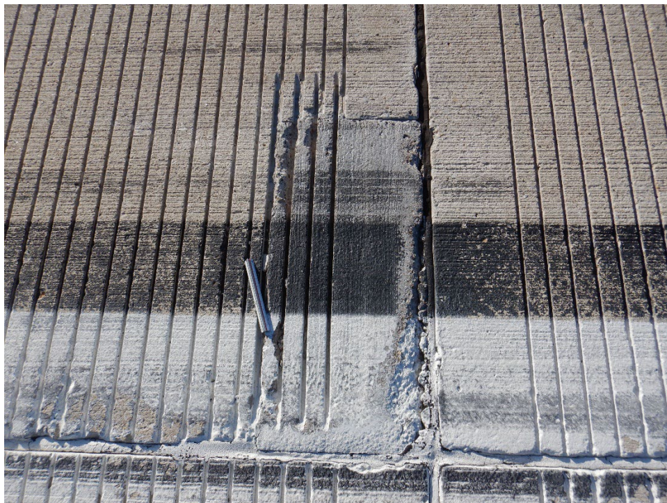
R07IC-01. Small Patching (Sample Unit No. 28).
