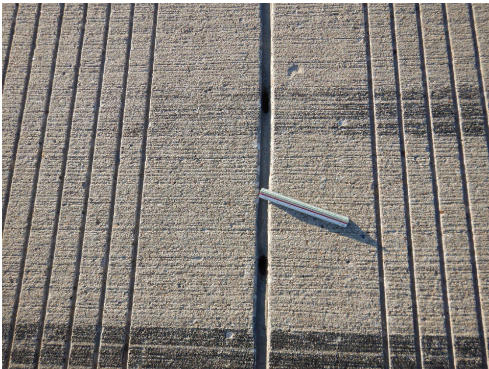
R07IC-02. Joint Seal Damage (Sample Unit No. 05).
