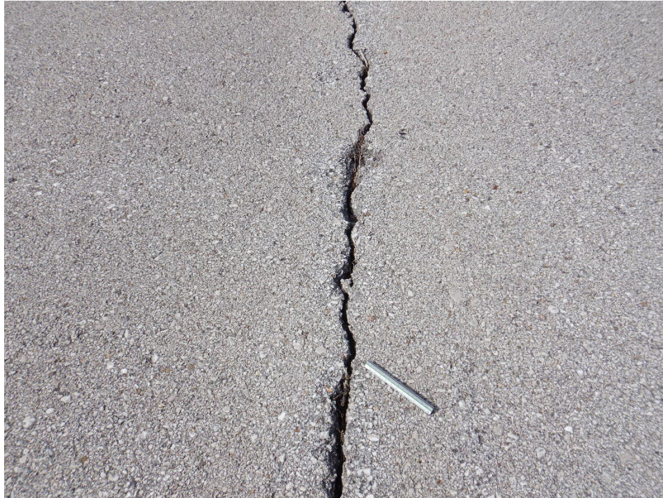
TBIC-04. L&T Cracking (Sample Unit No. 01) (2).
