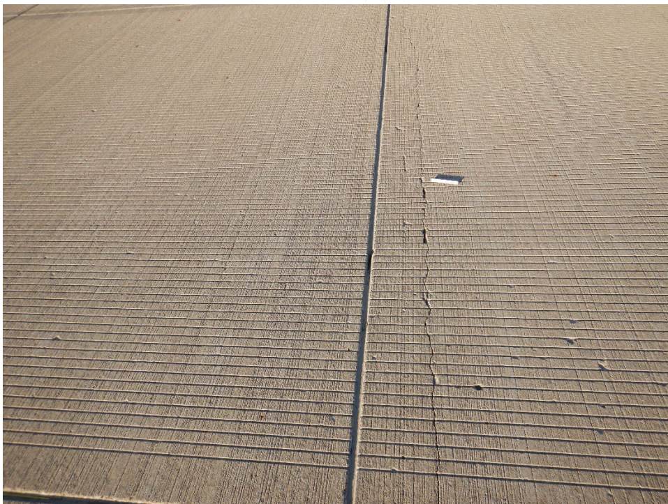
R07IC-03. LTD Cracking (Sample Unit No. 16) (3).
