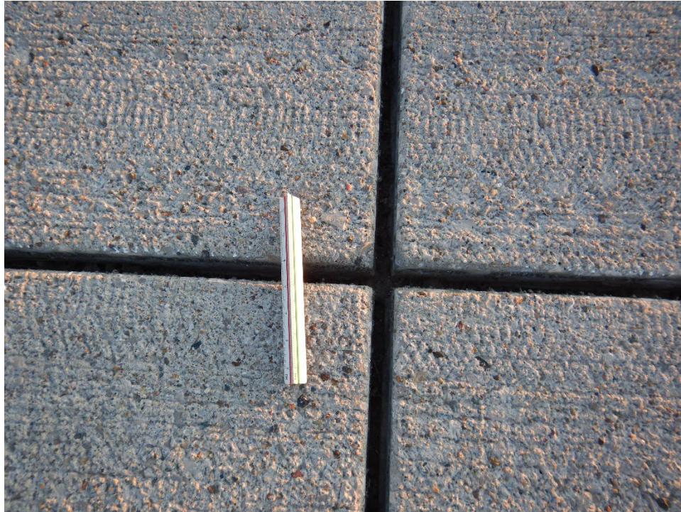
R12IC-01. Joint Seal Damage (Sample Unit No. 45).
