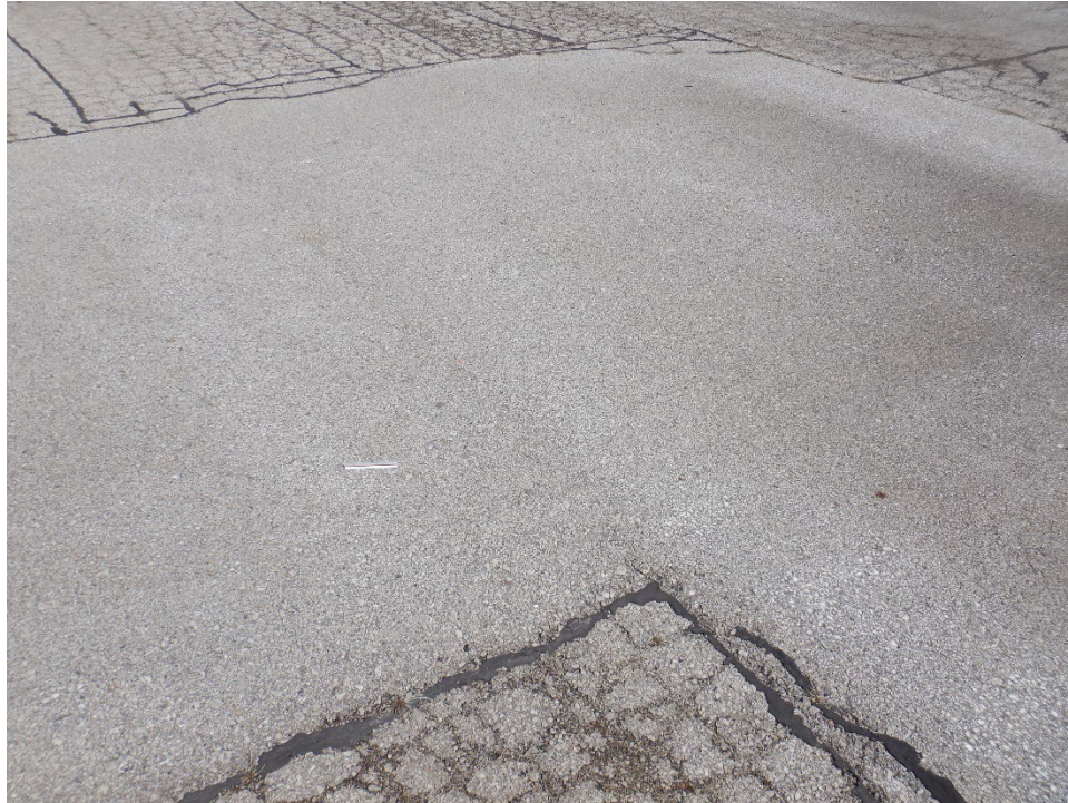
TH01IC-04. Patching (Sample Unit No. 17).
