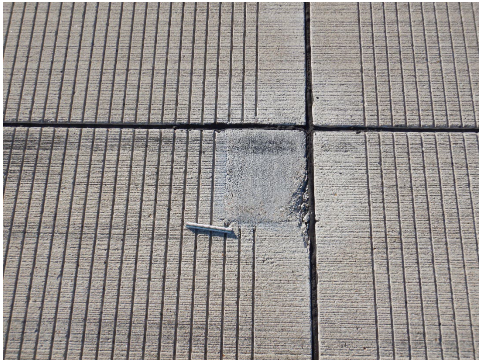
R07IC-01. Small Patching (Additional Sample Unit No. 36) (2).
