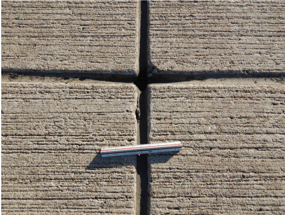
TAIC-01. Joint Seal Damage (Sample Unit No. 04).
