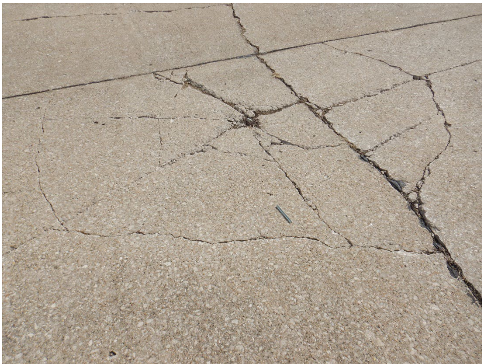
TH01IC-03. Shattered Slab (Sample Unit No. 02).
