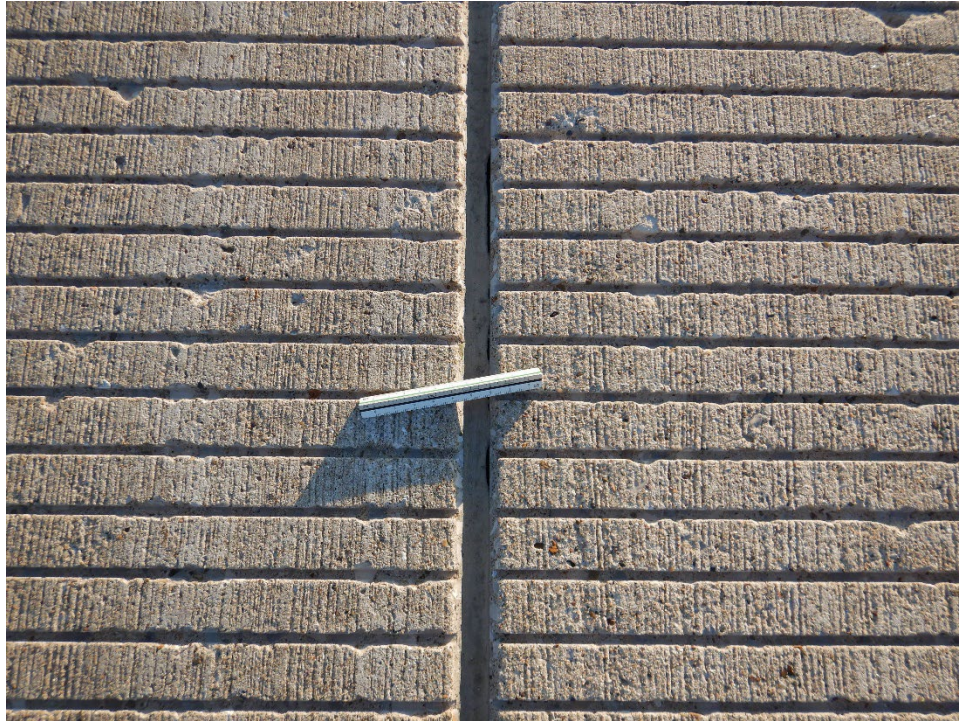
R07IC-03. Joint Seal Damage (Sample Unit No. 03).
