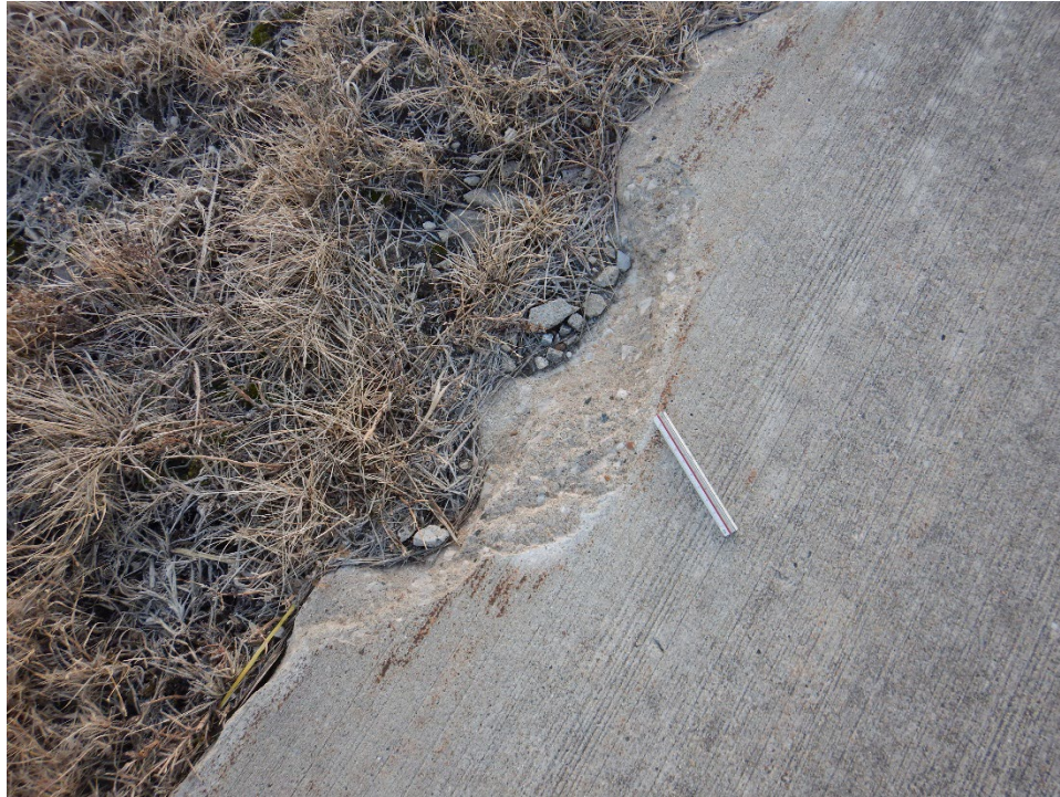
R12IC-01. Joint Spalling (Sample Unit No. 75).
