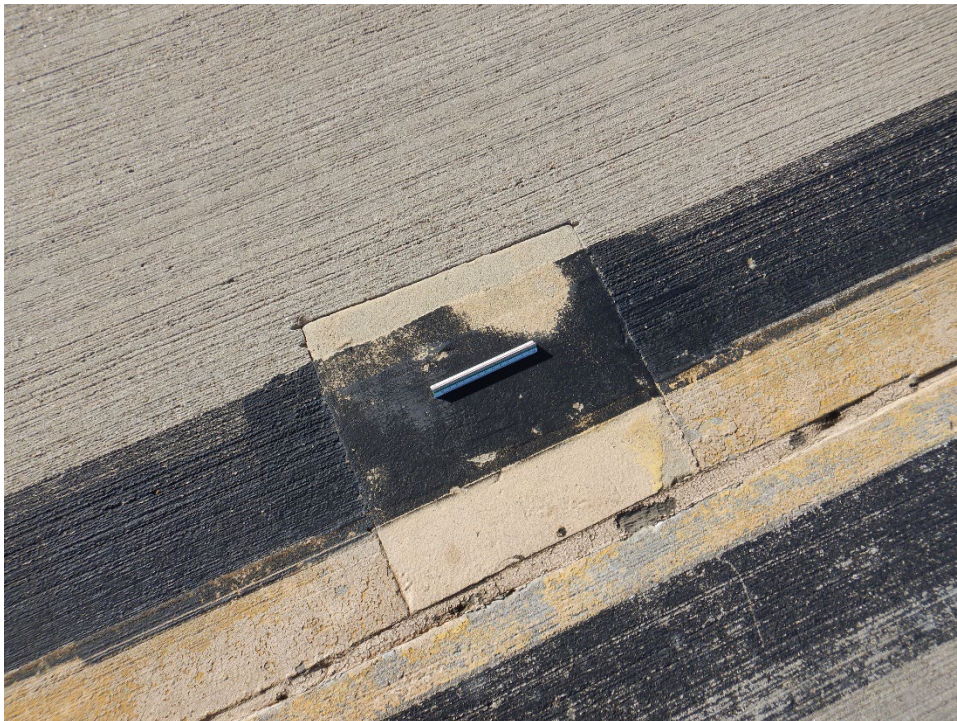
TH01IC-01. Small Patching (Sample Unit No. 04) (1).
