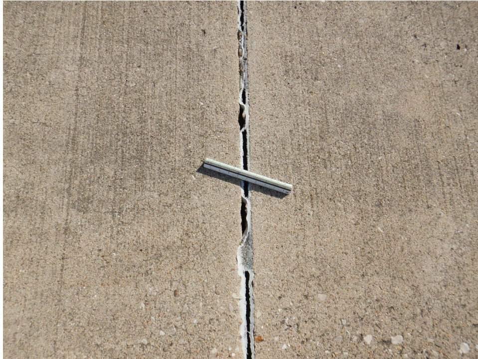
TH02IC-02. Joint Seal Damage (Sample Unit No. 14).
