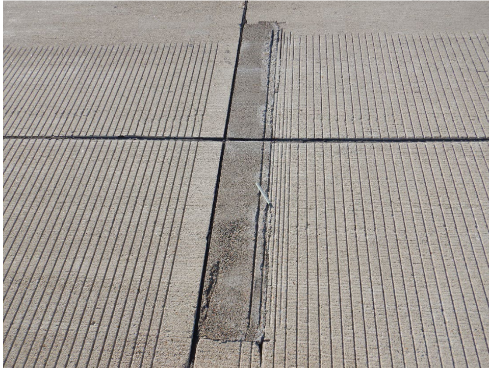
R07IC-01. Small Patching (Additional Sample Unit No. 36) (1).
