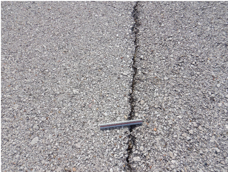
TBIC-04. L&T Cracking (Sample Unit No. 01) (1).
