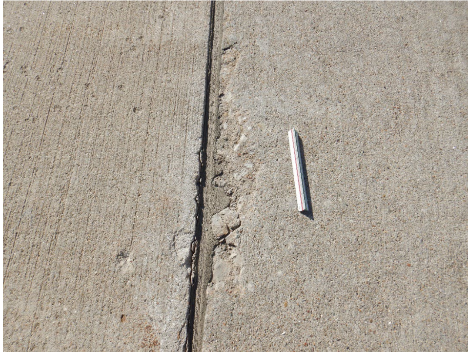
TH02IC-04. Joint Spalling (Sample Unit No. 02).
