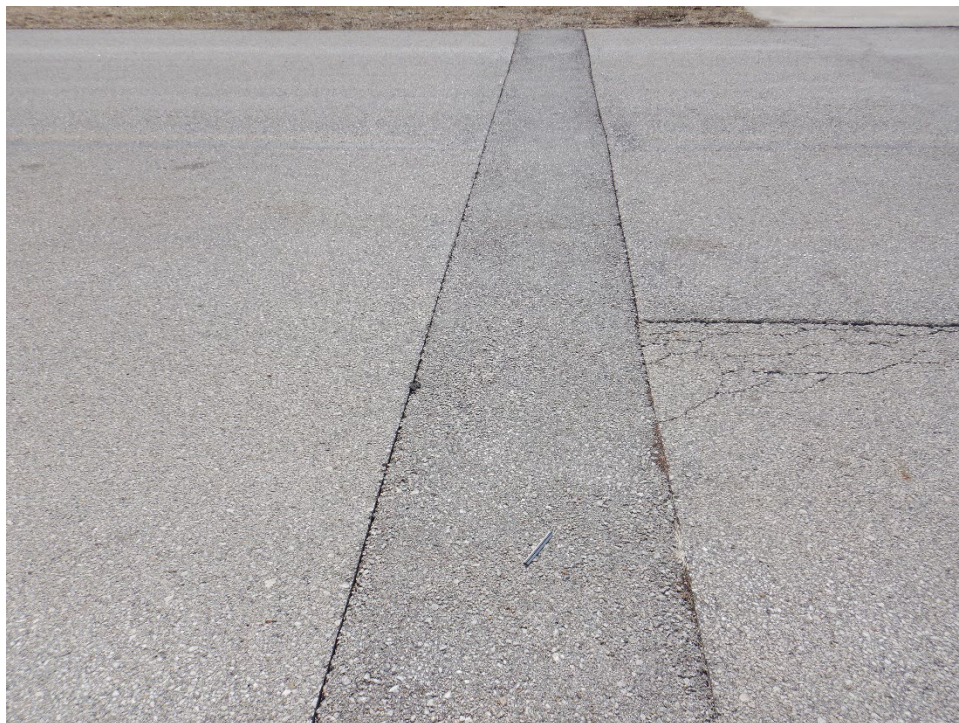
TH02IC-01. Patching (Sample Unit No. 01).
