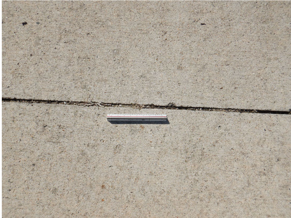
TH02IC-03. Joint Seal Damage (Sample Unit No. 01).
