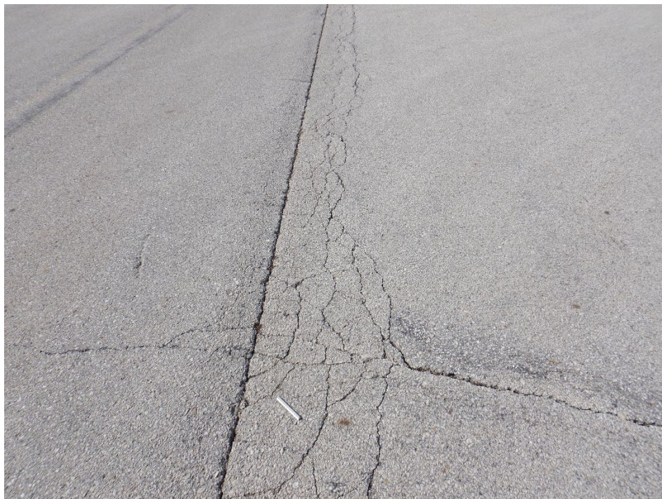
TH02IC-01. Alligator Cracking (Sample Unit No. 01) (2).
