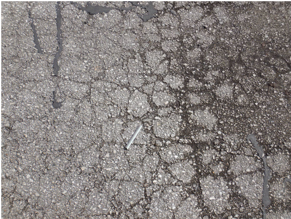
TH01IC-04. Alligator Cracking (Sample Unit No. 17).
