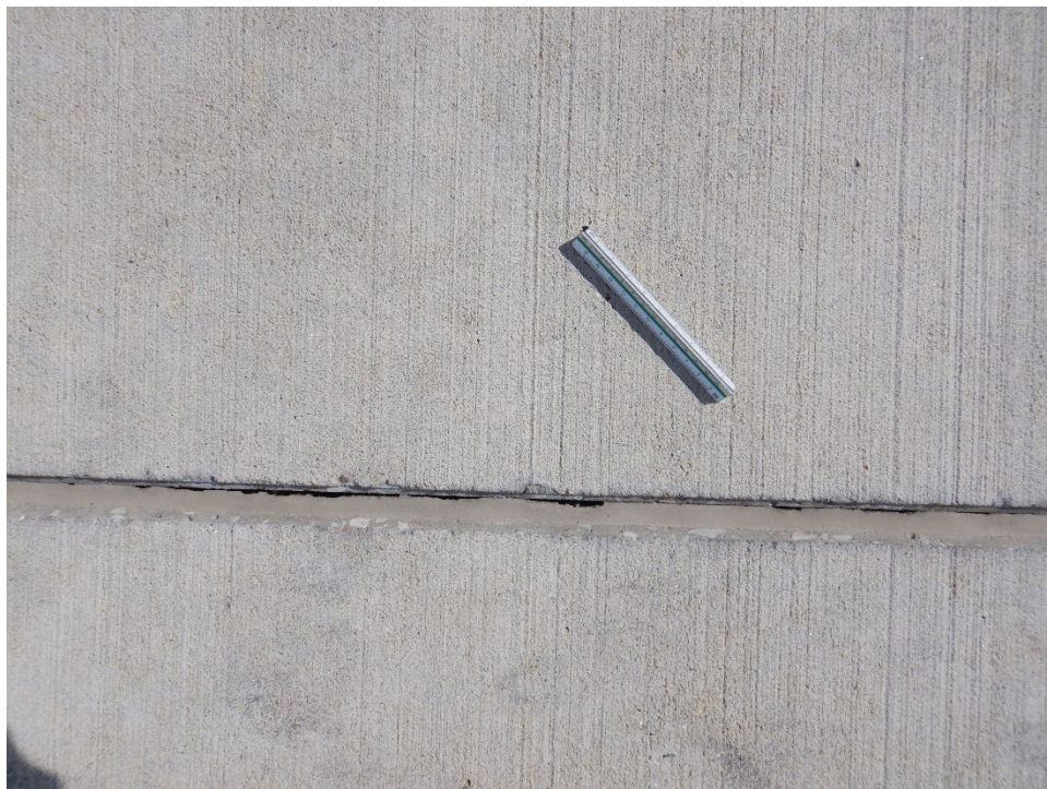
A01IC-01. Joint Seal Damage (Sample Unit No. 08).
