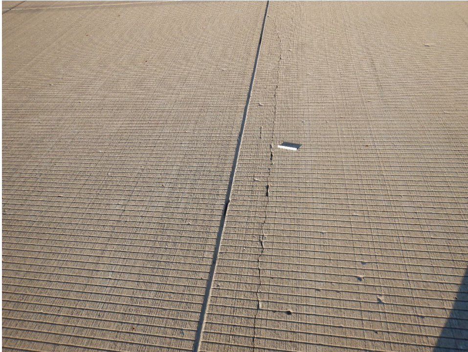
R07IC-03. LTD Cracking (Sample Unit No. 16) (2).
