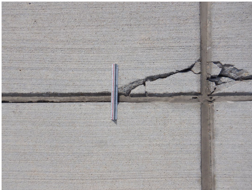
TBIC-02. Joint Spalling (Sample Unit No. 02).
