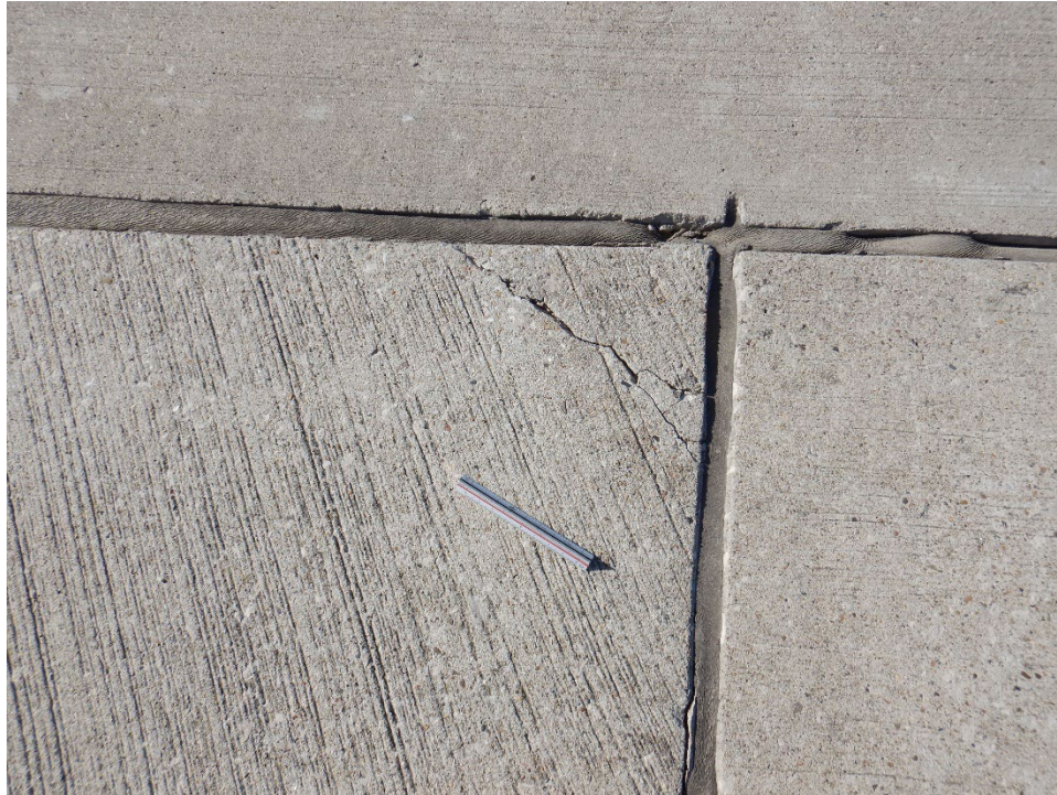
TBIC-06. Corner Spalling (Sample Unit No. 04).
