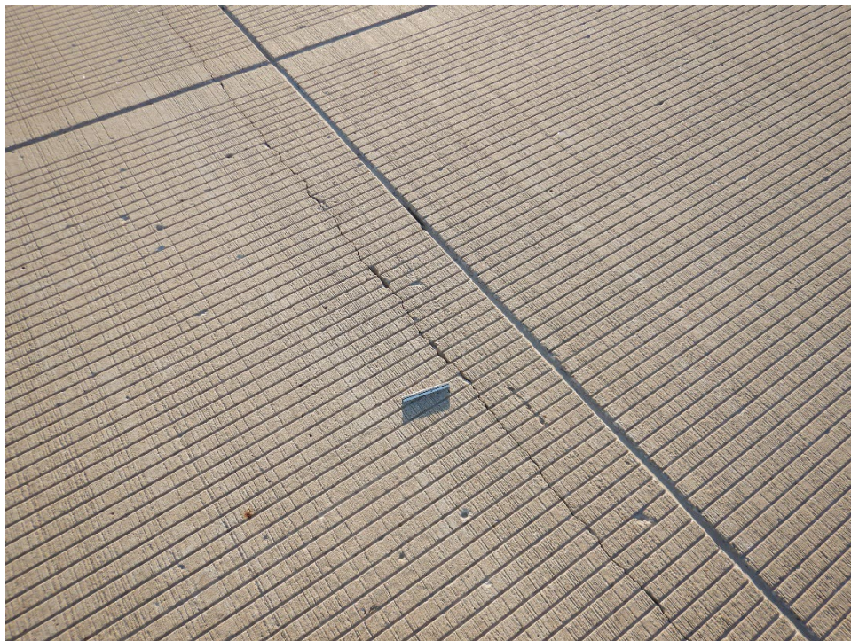
R07IC-03. LTD Cracking (Sample Unit No. 16) (1).
