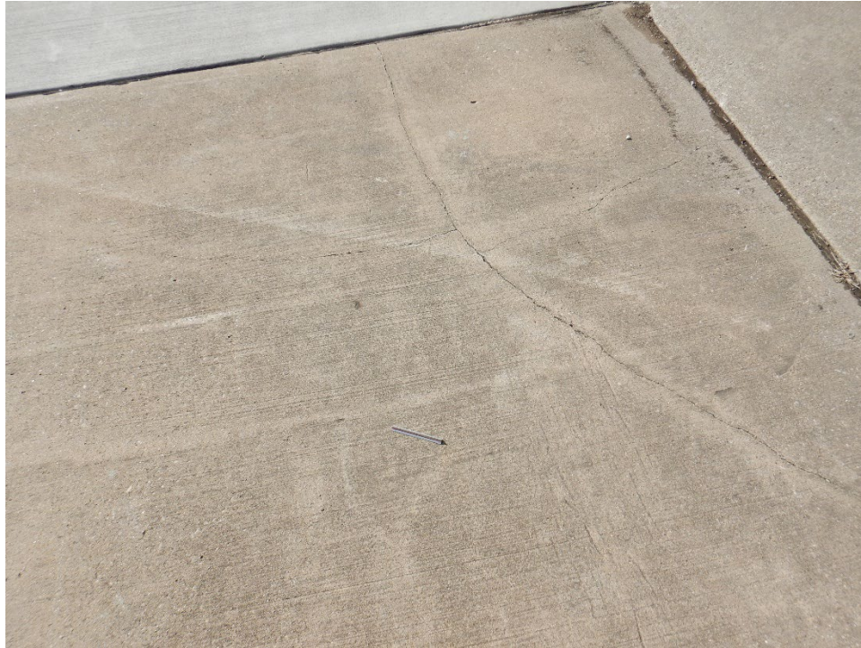
TH02IC-02. Shattered Slab (Sample Unit No. 14).
