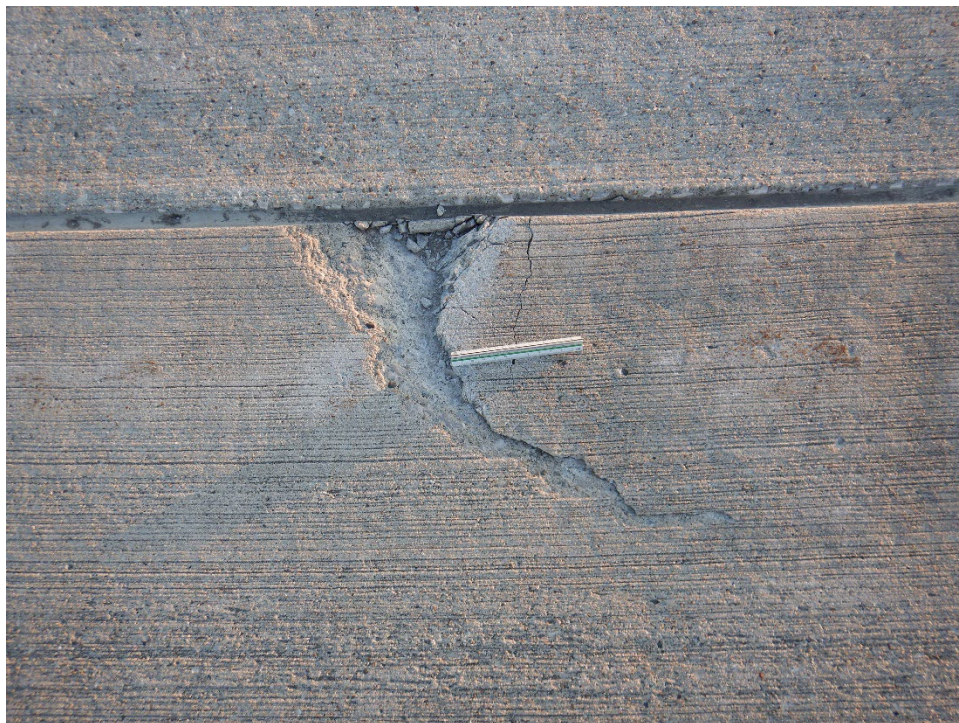
R12IC-01. Joint Spalling (Sample Unit No. 35).
