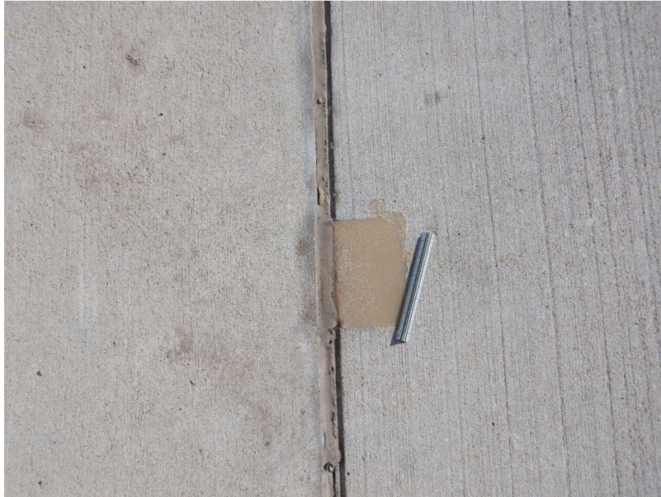
A01IC-01. Small Patching (Sample Unit No. 06).
