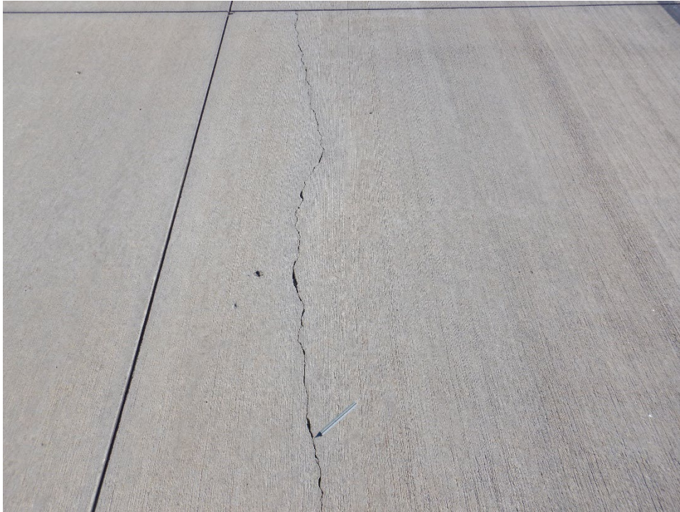
TAIC-02. LTD Cracking (Additional Sample Unit No. 090).
