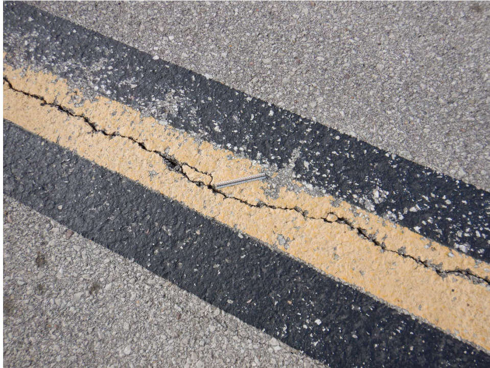
TBIC-01. Joint Reflection Cracking (Sample Unit No. 01).
