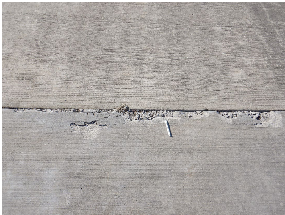
TBIC-06. Joint Spalling (Additional Sample Unit No. 01).
