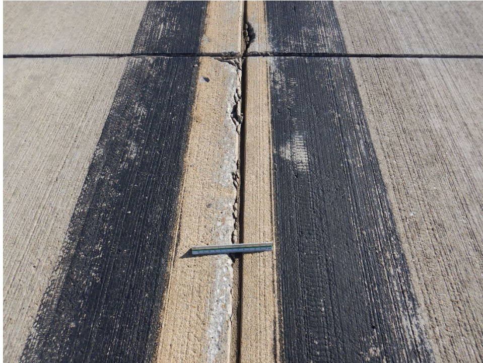
TAIC-02. Joint Seal Damage (Additional Sample Unit No. 089).
