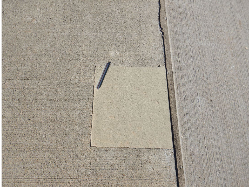
TH01IC-01. Small Patching (Sample Unit No. 04) (2).
