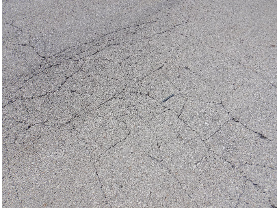
TH02IC-01. Alligator Cracking (Sample Unit No. 03).
