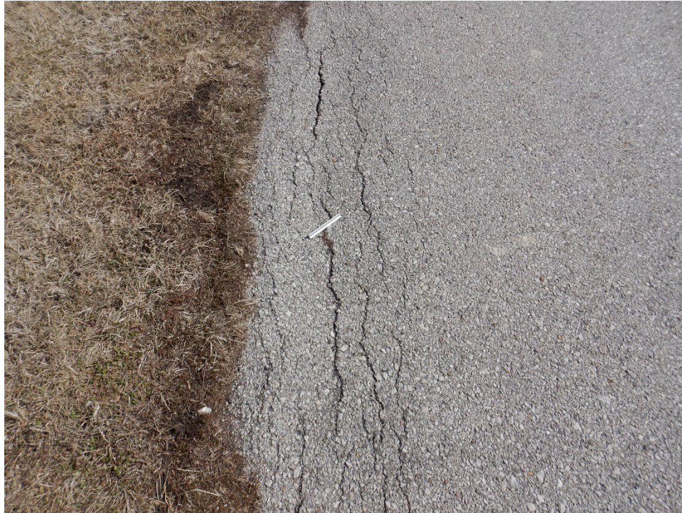
TH02IC-01. Alligator Cracking (Sample Unit No. 01) (1).
