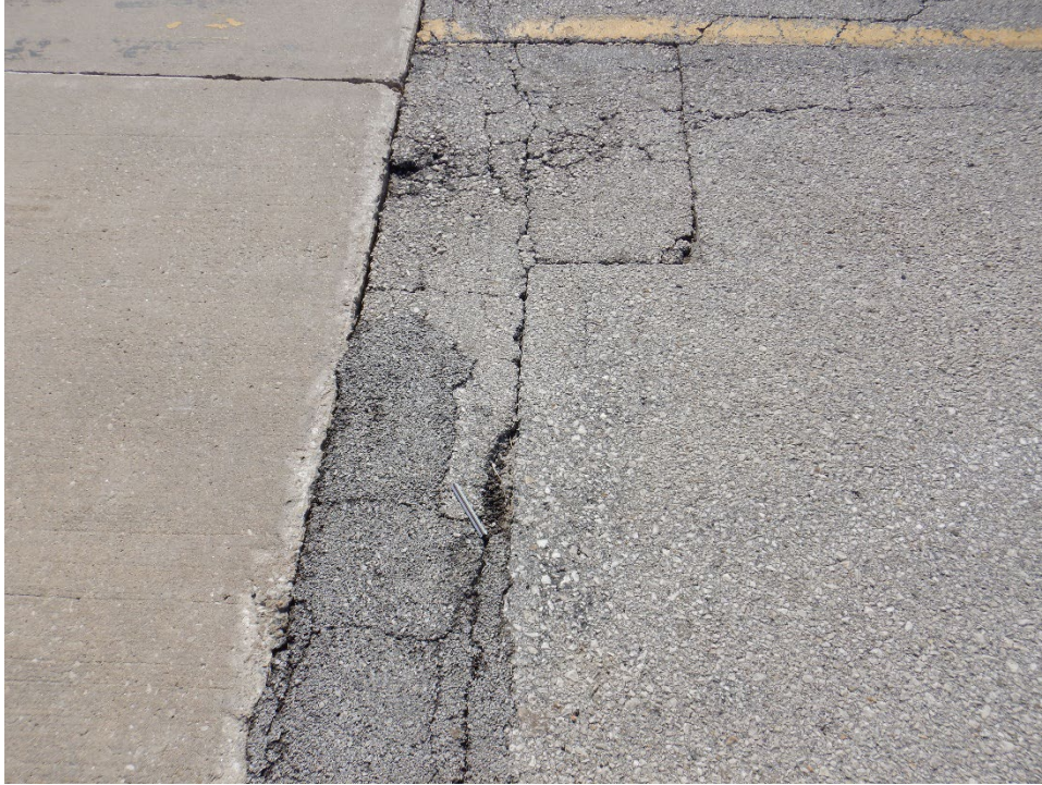
TH02IC-01. Patching (Sample Unit No. 03).
