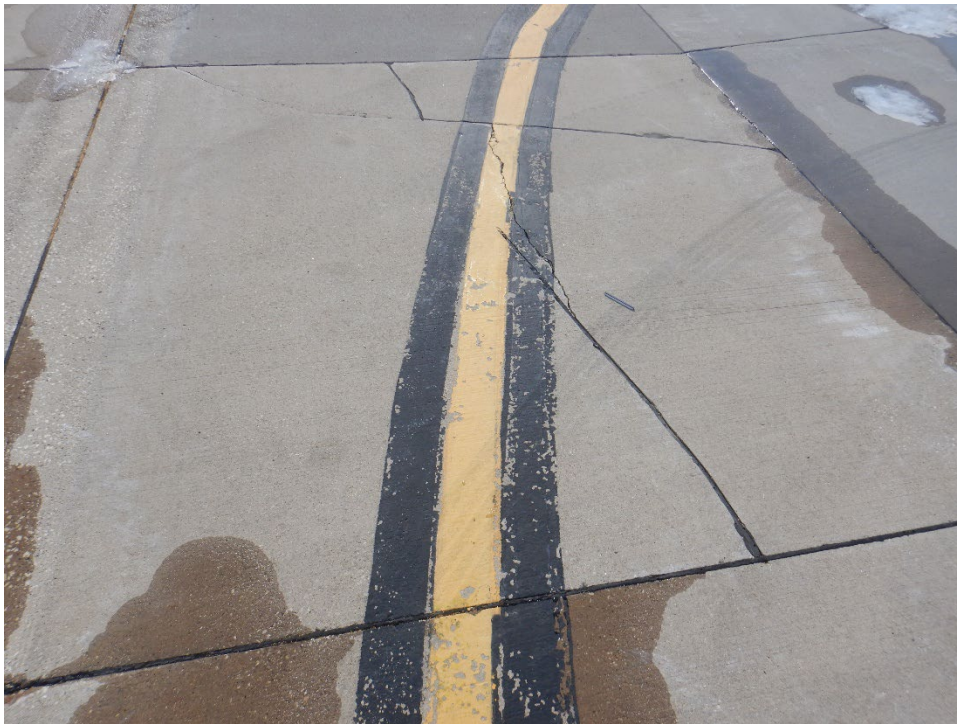
TH01IN-02. Shattered Slab (Sample Unit No. 03).
