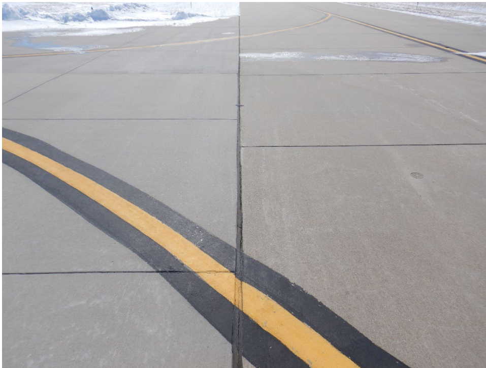
T04IN-01. Faulting (Additional Sample Unit No. 01).
