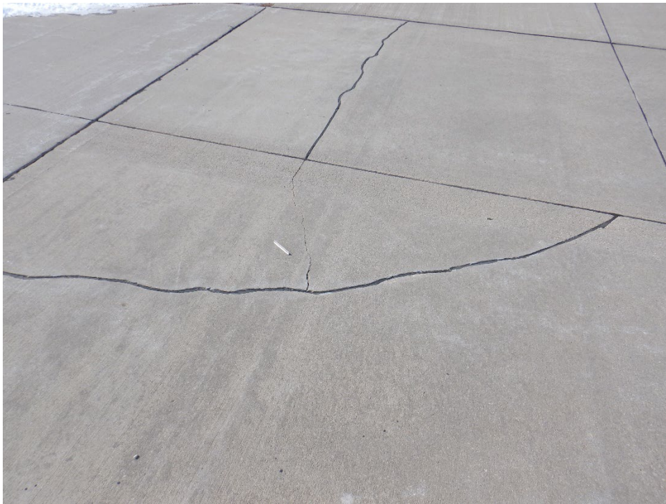
TH01IN-03. LTD Cracking (Sample Unit No. 02).
