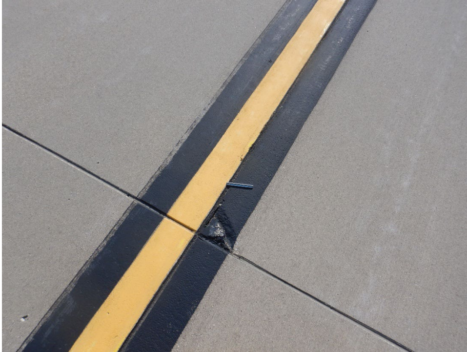
TAIN-01. Corner Spalling (Sample Unit No. 100).
