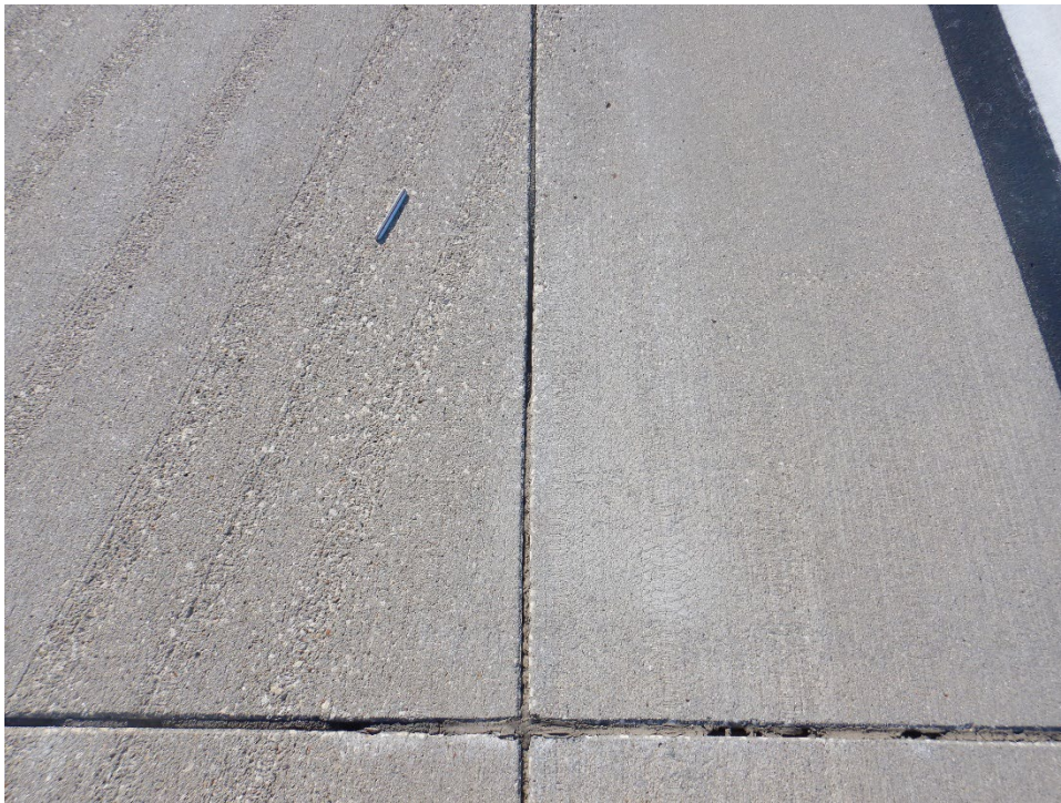
R18IN-02. Joint Seal Damage (Sample Unit No. 33).
