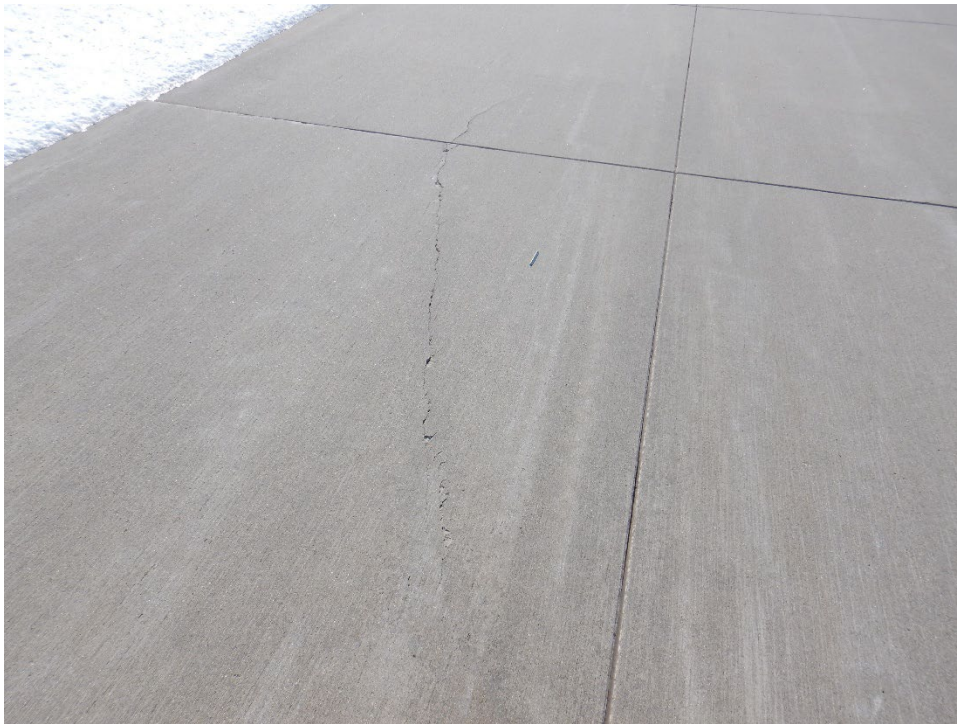
R18IN-01. LTD Cracking (Additional Sample Unit No. 55).
