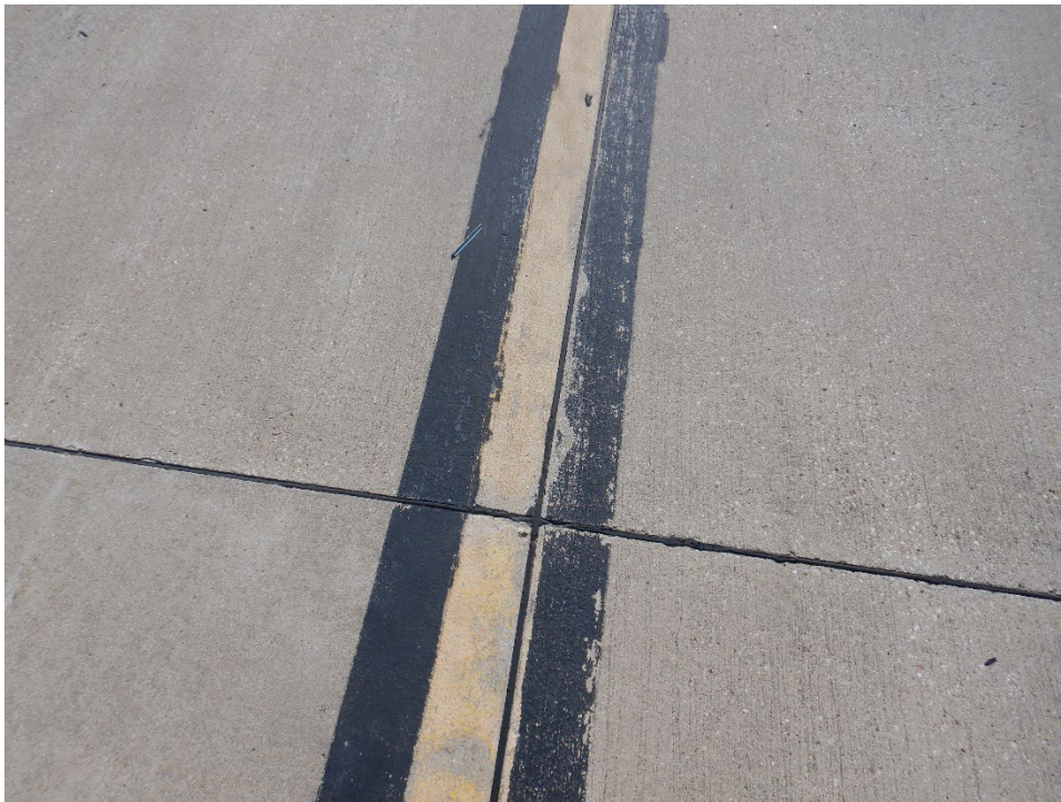
TH01IN-01. Joint Seal Damage (Sample Unit No. 03).
