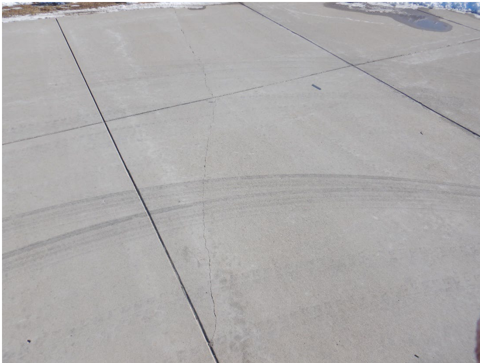
T03IN-01. LTD Cracking (Sample Unit No. 12).
