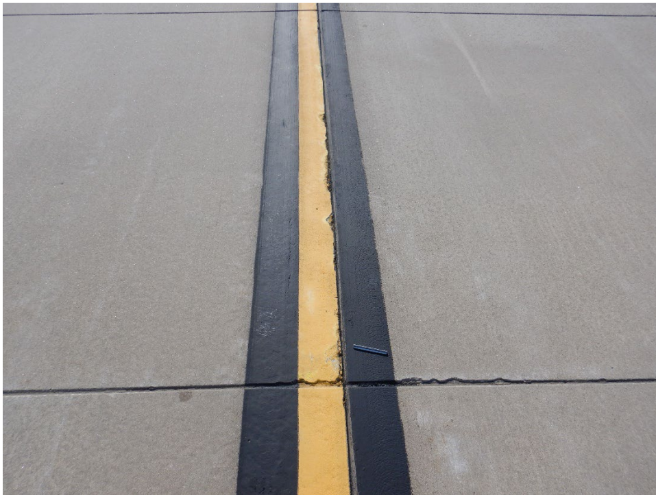
TAIN-01. Joint Seal Damage (Sample Unit No. 70).
