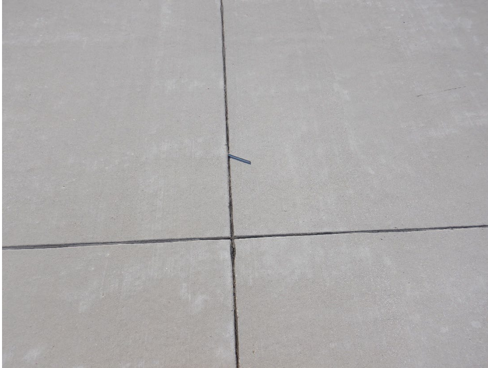
T04IN-01. Joint Seal Damage (Sample Unit No. 09).
