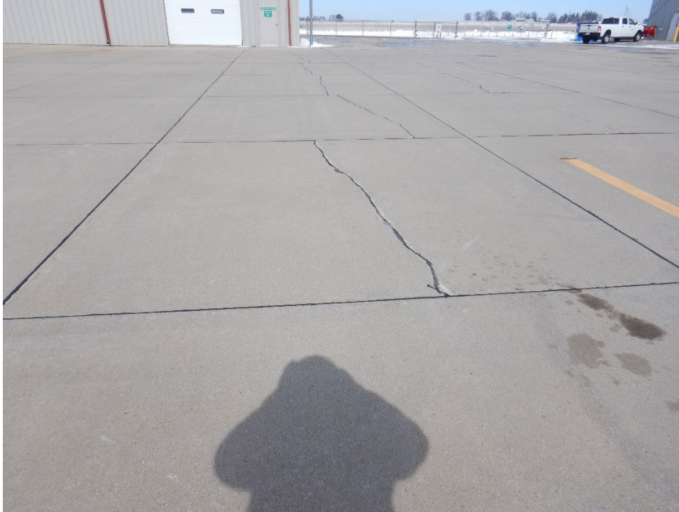
A01IN-01. LTD Cracking (Sample Unit No. 08).
