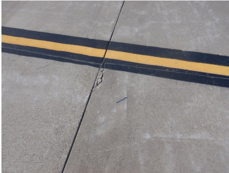
TA3IN-01. Joint Spalling (Sample Unit No. 09).
