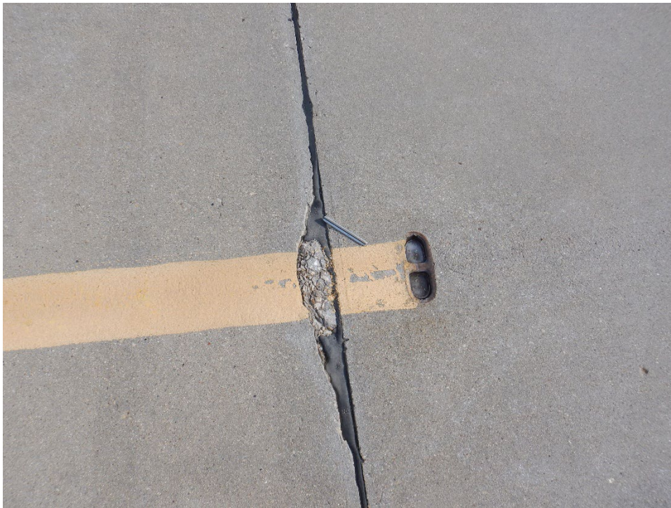
A01IN-01. Joint Spalling (Sample Unit No. 08).
