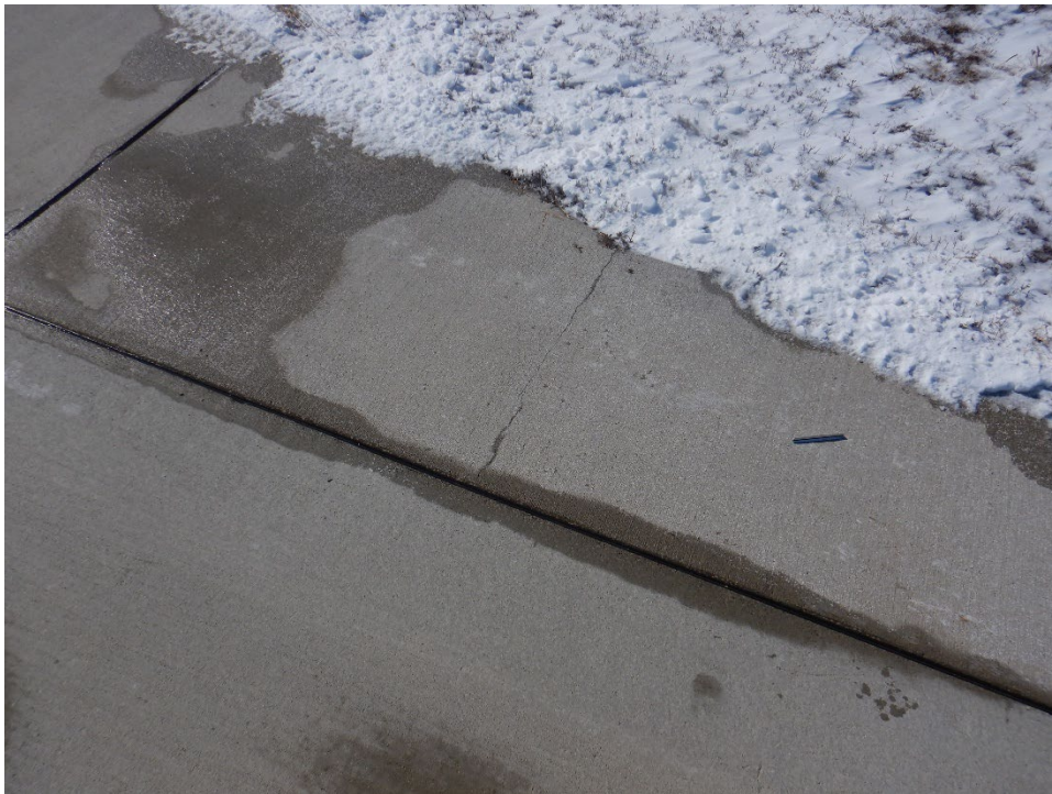
A02IN-01. LTD Cracking (Sample Unit No. 04).
