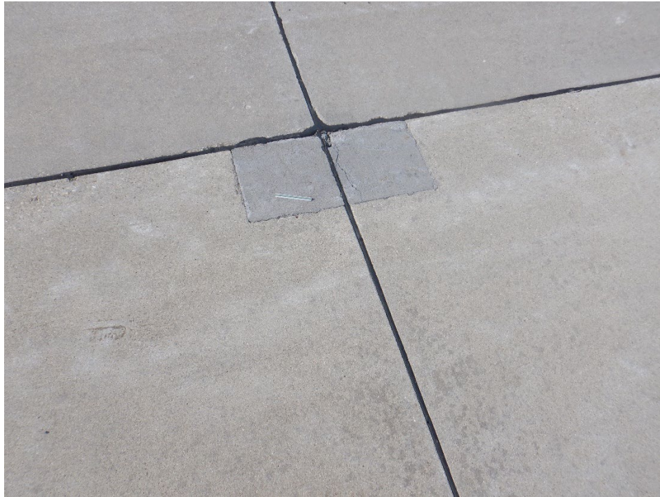
A01IN-02. Small Patching (Sample Unit No. 03).
