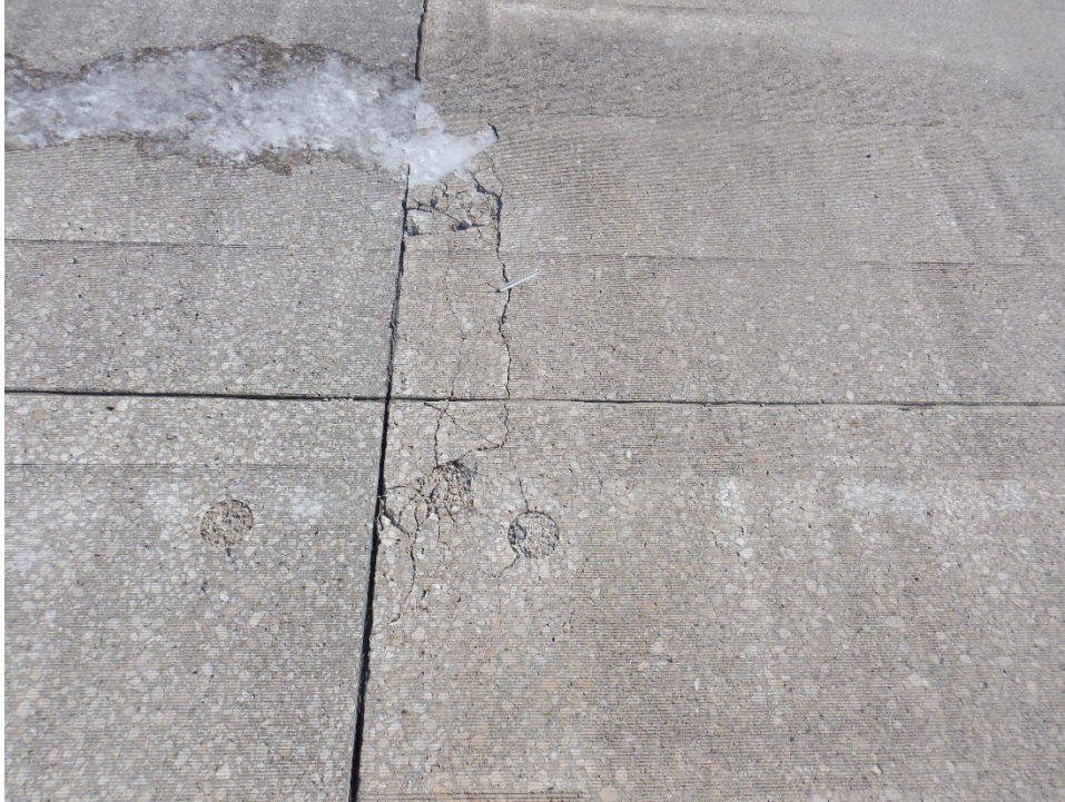
R18IN-01. Joint Spalling (Additional Sample Unit No. 01).
