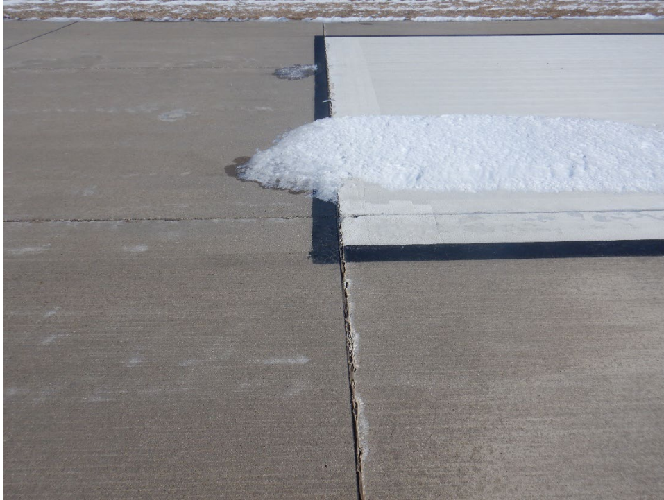
R18IN-02. Faulting (Additional Sample Unit No. 09).
