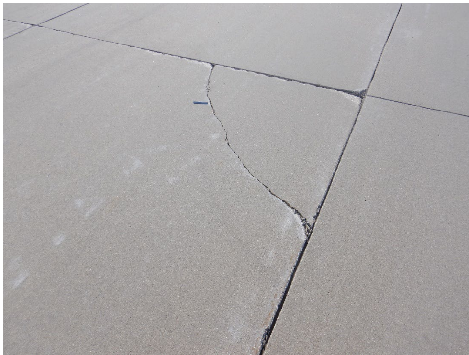
R18IN-02. Corner Break (Additional Sample Unit No. 22).
