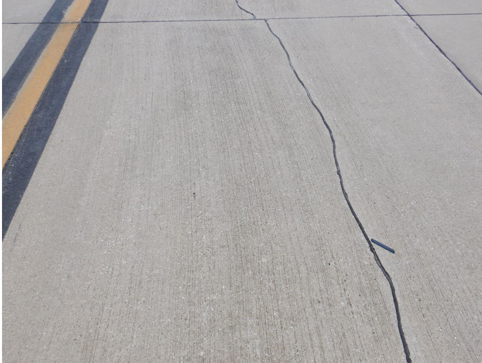
TH01IN-01. LTD Cracking (Sample Unit No. 03).
