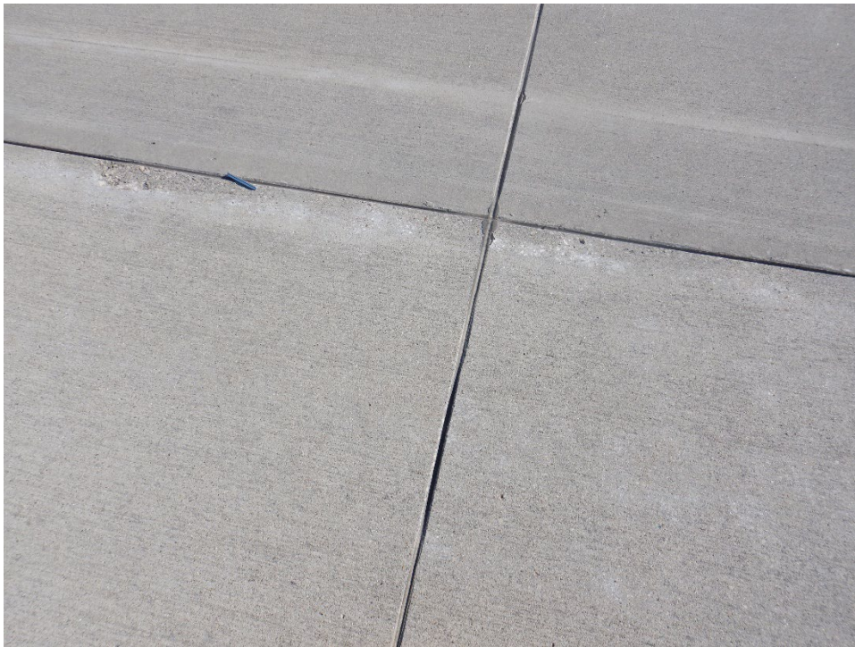
R18IN-01. Joint Seal Damage (Sample Unit No. 56).
