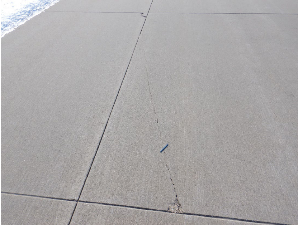
R18IN-02. LTD Cracking (Additional Sample Unit No. 26).
