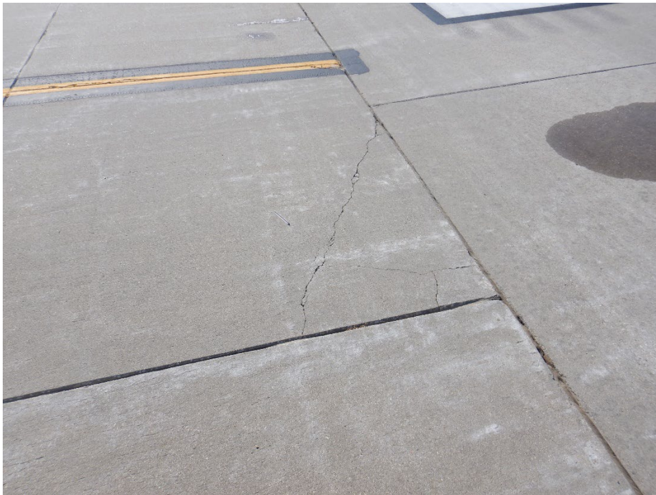
R18IN-02. LTD Cracking (Additional Sample Unit No. 41).
