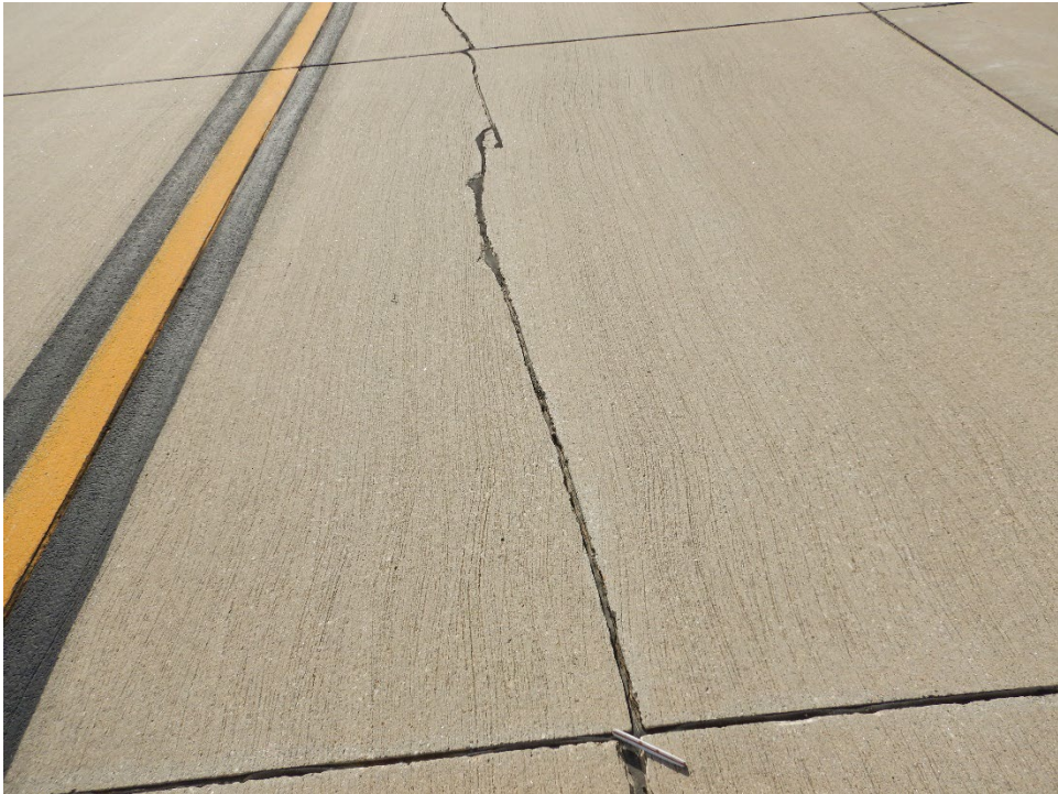
TH01IN-01. LTD Cracking (Sample Unit No. 02).
