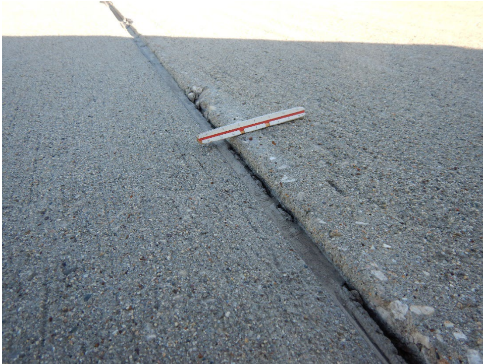
R18IN-01. Faulting (Sample Unit No. 22).
