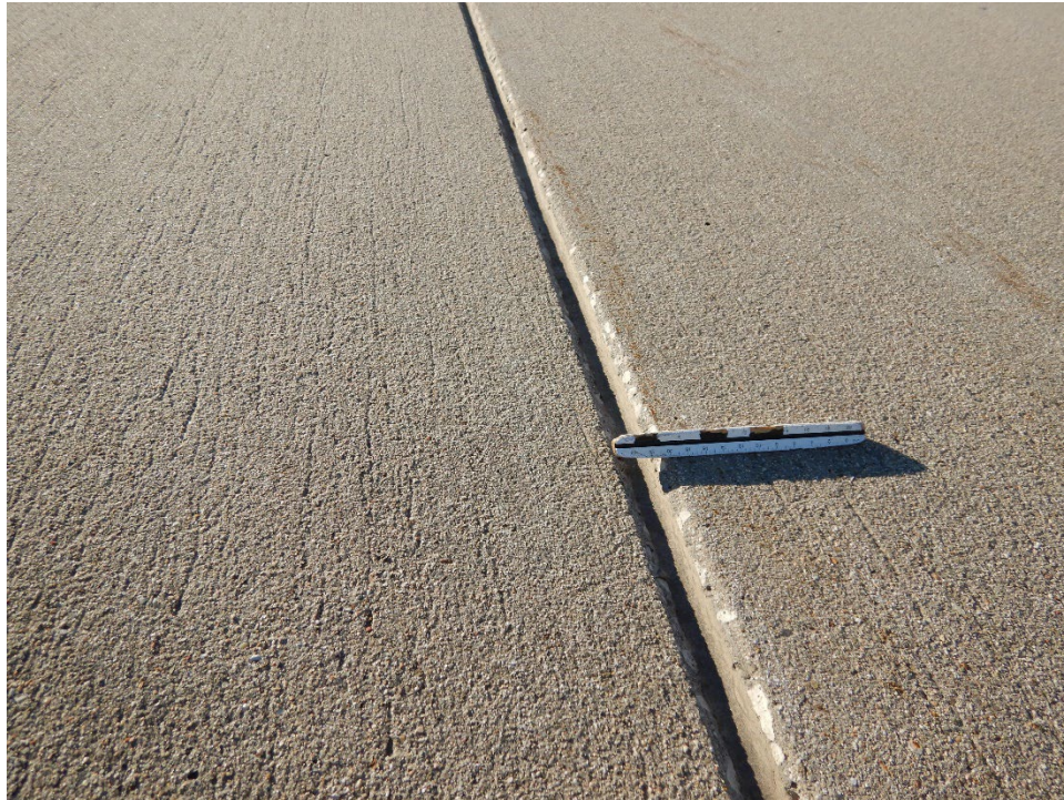
R18IN-02. Faulting (Sample Unit No. 03).
