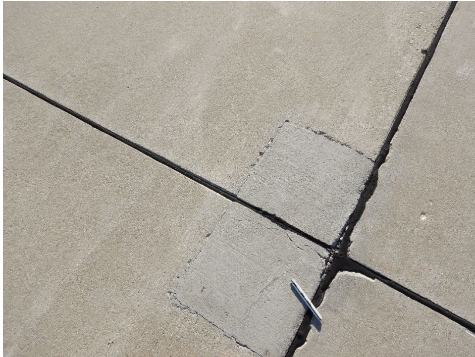
A01IN-02. Small Patching (Sample Unit No. 03).
