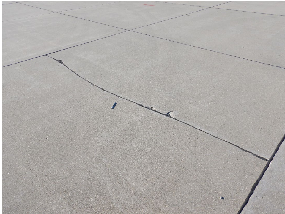
A01IN-01. LTD Cracking (Sample Unit No. 17).
