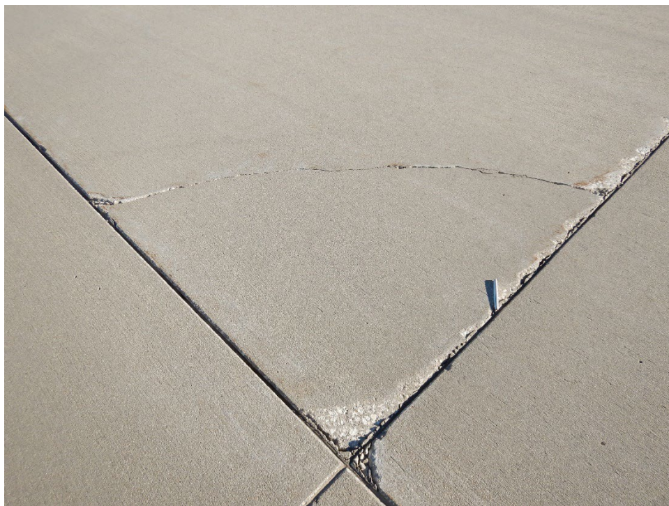
R18IN-02. Corner Break (Additional Sample Unit No. 22).
