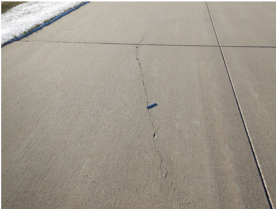
R18IN-01. LTD Cracking (Additional Sample Unit No. 055).
