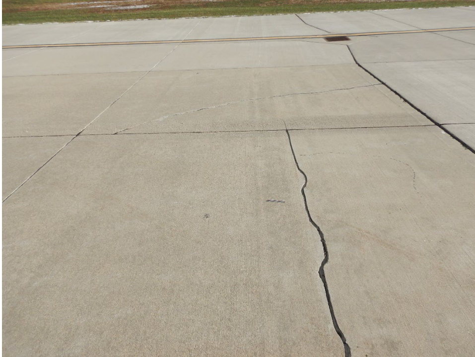
TH01IN-03. LTD Cracking (Sample Unit No. 02).
