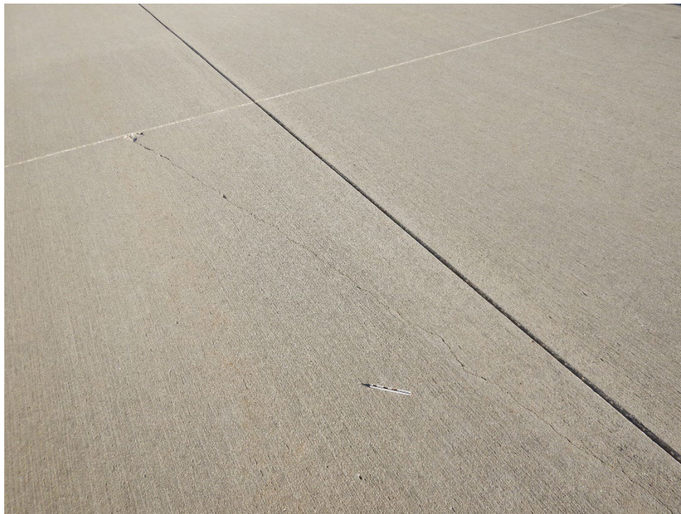
R18IN-02. LTD Cracking (Additional Sample Unit No. 24).
