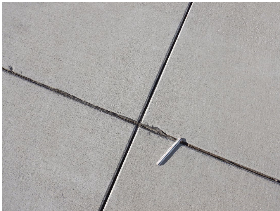
T03IN-01. Joint Seal Damage (Sample Unit No. 12).
