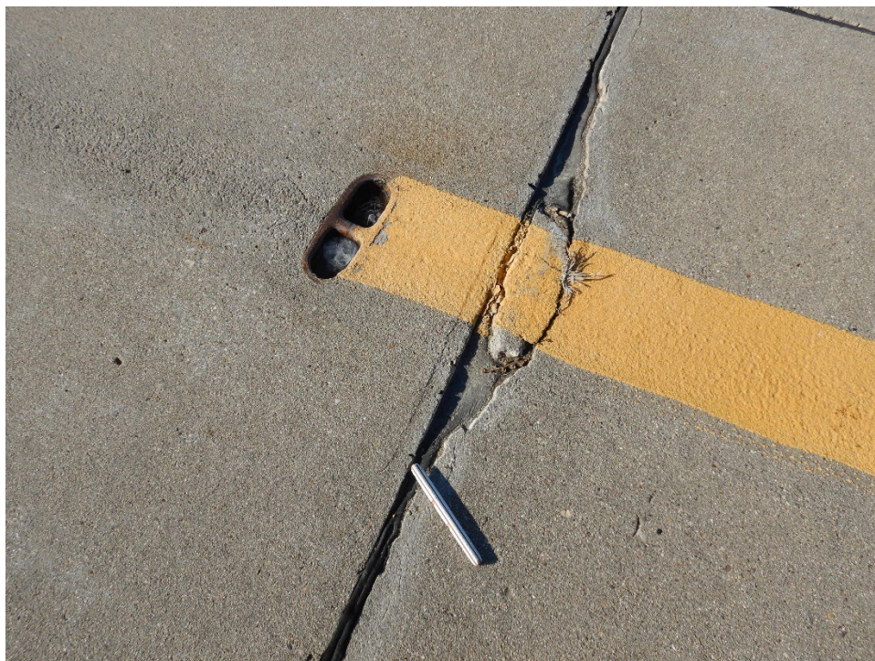
A01IN-01. Joint Spalling (Sample Unit No. 08).
