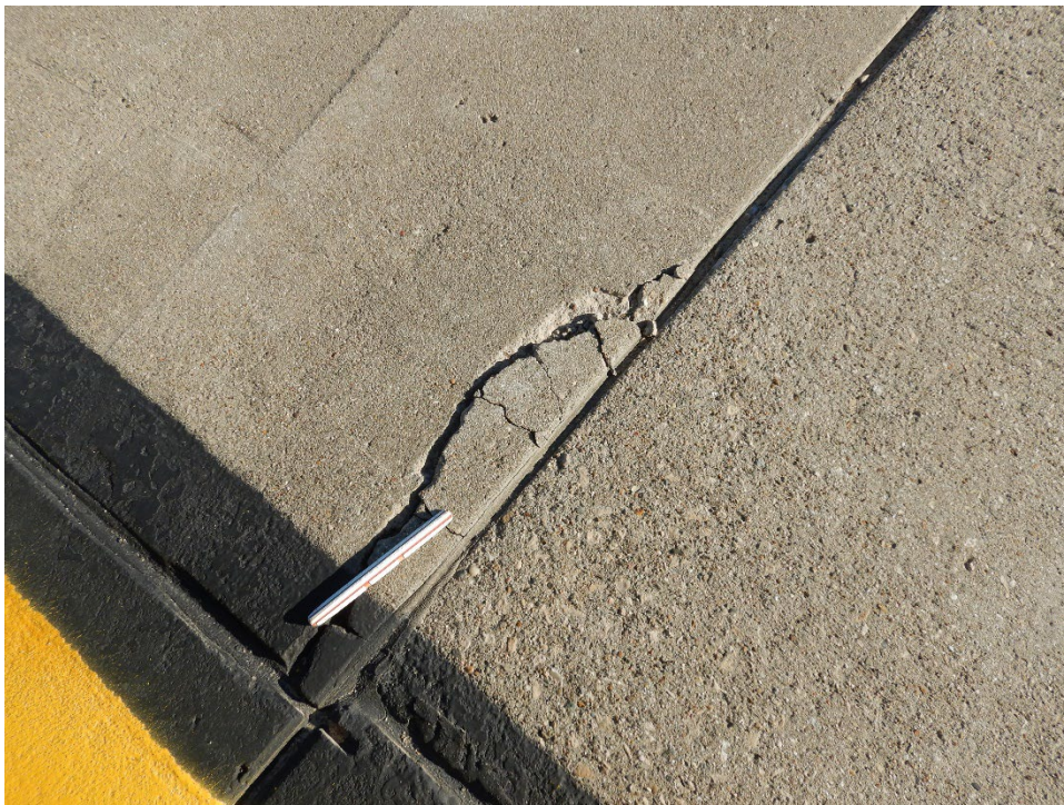
T01IN-01. Joint Spalling (Sample Unit No. 09).
