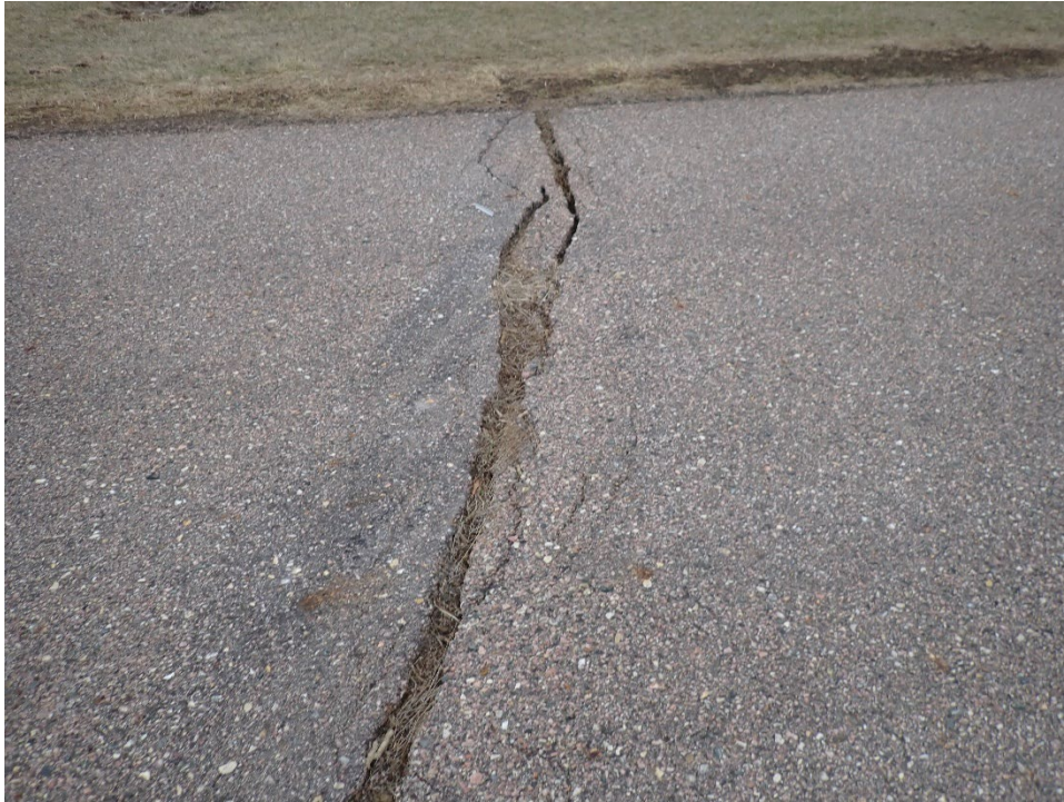
R12IG-01. L&T Cracking (Sample Unit No. 03).
