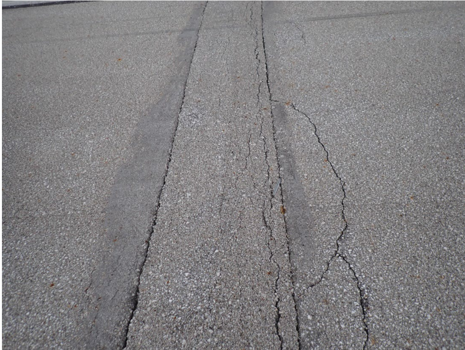
R12IG-02. Patching (Sample Unit No. 05).
