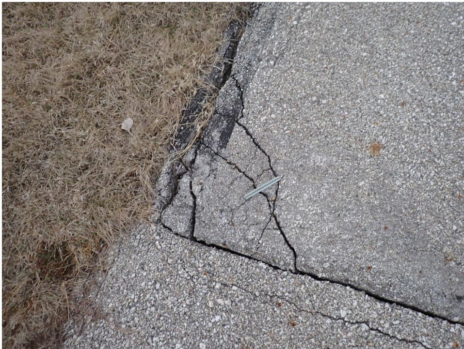
R12IG-02. Alligator Cracking (Sample Unit No. 05).
