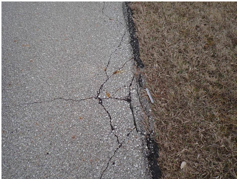
R12IG-03. Alligator Cracking (Sample Unit No. 01).
