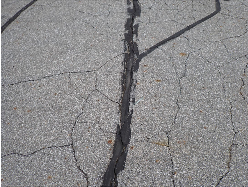
T01IG-01. Alligator Cracking (Sample Unit No. 03) (2).
