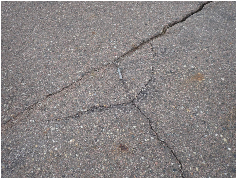
R12IG-01. Alligator Cracking (Sample Unit No. 04).
