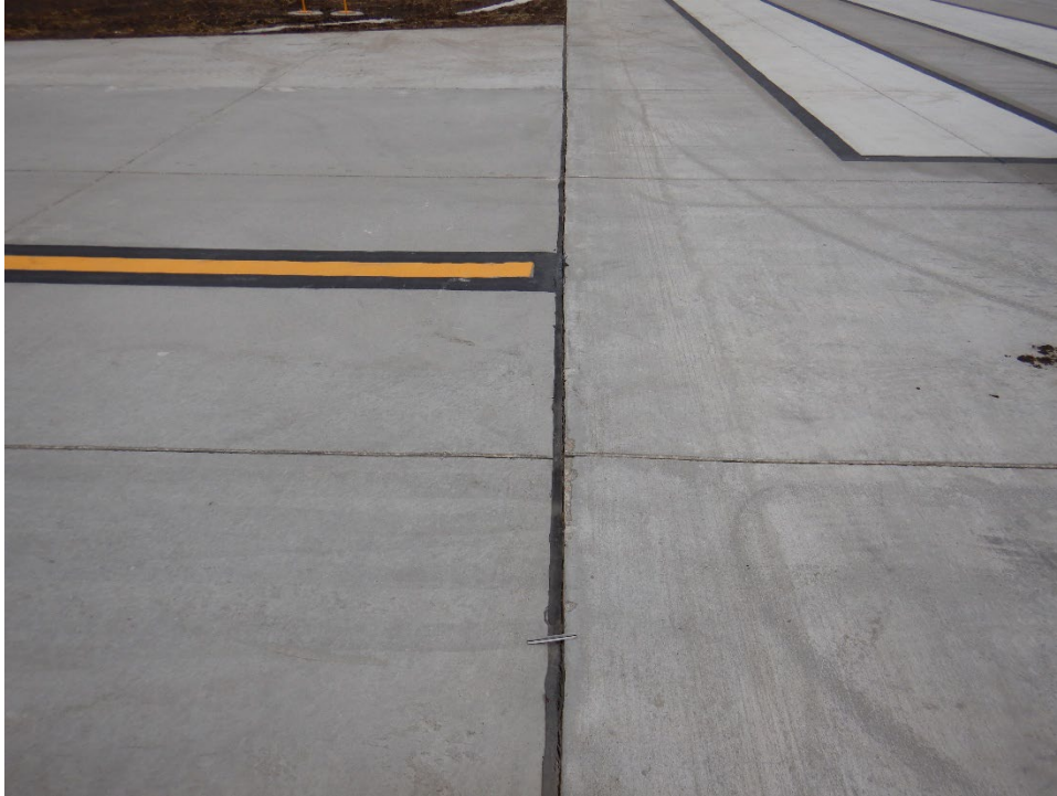
R12HU-02. Faulting (Additional Sample Unit No. 17).
