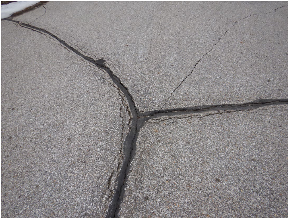
A01HU-01. L&T Cracking (Sample Unit No. 01).
