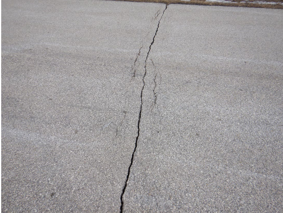
TH01HU-01. L&T Cracking (Sample Unit No. 01).
